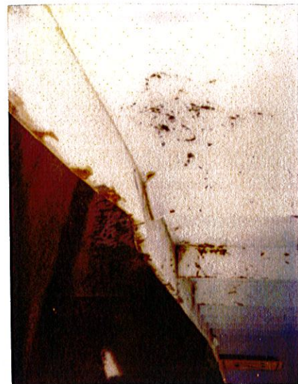
Bm #1 Outside Bent Stiffener Bent Bottom Flange
