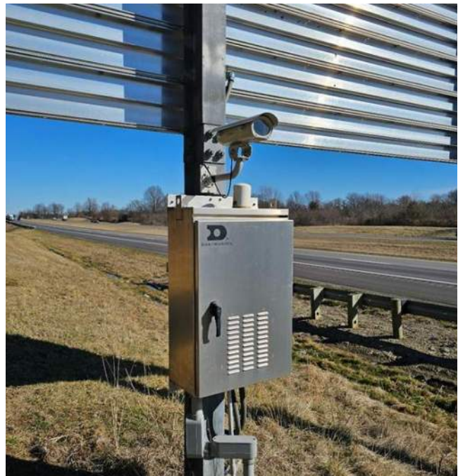
Figure 13: QWS-D5-I-70_WB Existing detection camera on back of existing DDMS
