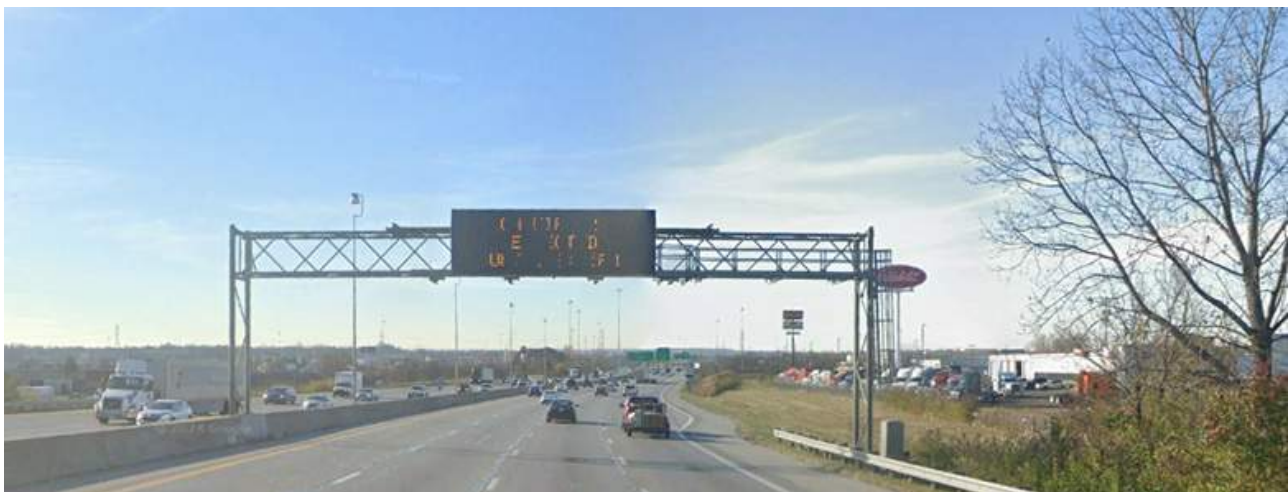
Figure 50: QWS-OVRHD-D8-I-275_WB AT I-75 NB existing DMS to be replaced
