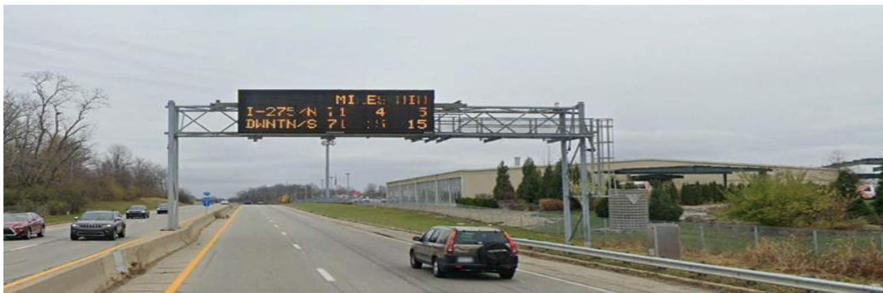
Figure 46: QWS-OVRHD-D8-OH-126_EB AT I-71 existing DMS to be replaced
