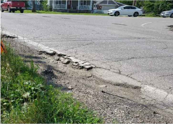
Photo 1: Broken Pavement on Shoulder
