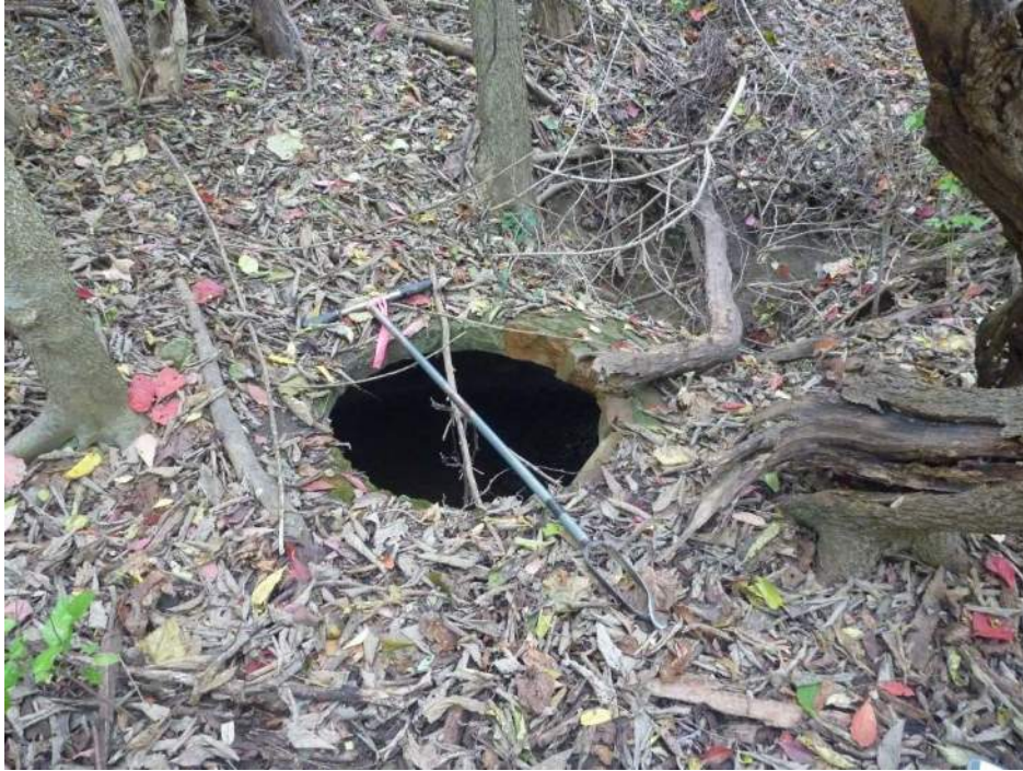
Photo Location 12: Abandoned well, facing northwest.
