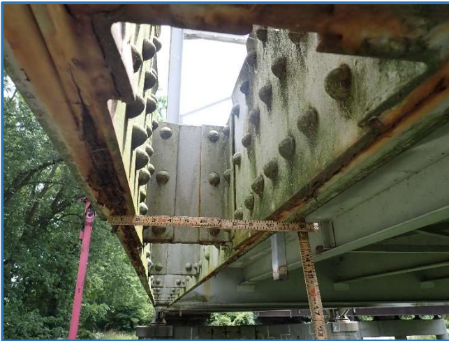
Photo 15 - 3/4" pack rust in lower chord plates in Span 3, North Truss, member L7L8, looking east
