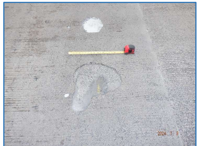
Photo 5 - Spalls in wearing surface on Span 3, left lane, between Panel Points 2 and 3
