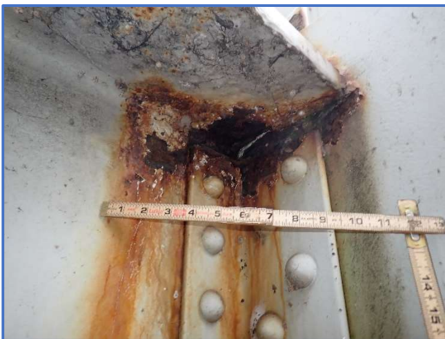
Photo 52 - Corrosion along top flange and clip angle in Span 1, Floorbeam 6 west face, north end, looking north
