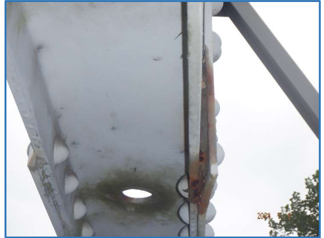
Photo 73 - Bowing of lower sway bracing connection plate due to pack rust in Span 3 at Panel Point 4, looking north
