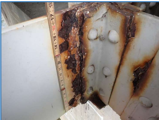
Photo 24 - Active laminar corrosion throughout the connection, Span 2, North Truss, at Panel Point 0, looking west
