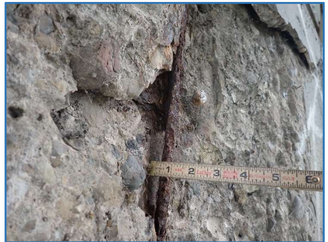
Photo 75 - Spall in west face of Pier 2 with exposed debonded rebar under Stringer 5
