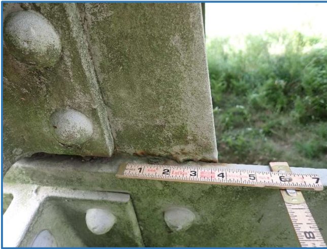
Photo 20 - Broken tack weld between lower chord and gusset plates, Span 4, North Truss, at Panel Point 1, looking south
