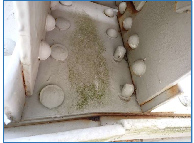
Photo 29 – Typical improperly installed rivet heads in stiffener plate, Span 3, North Truss, at Panel Point 3
