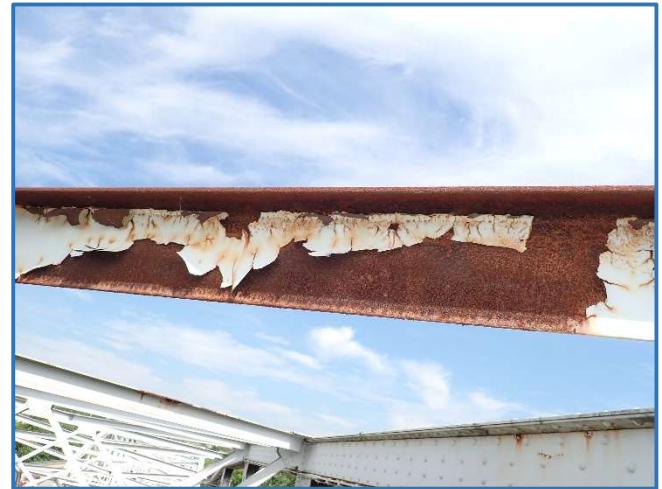
Photo 70 - Paint failure with surface corrosion on upper lateral brace in Span 3, between Panel Points 5 and 6, looking northwest
