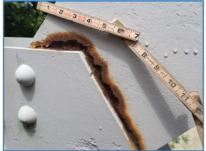
Photo 45 - 3/16" deep section loss along lower gusset plate on south face of diagonal in Span 2, North Truss, at Panel Point 8, looking north
