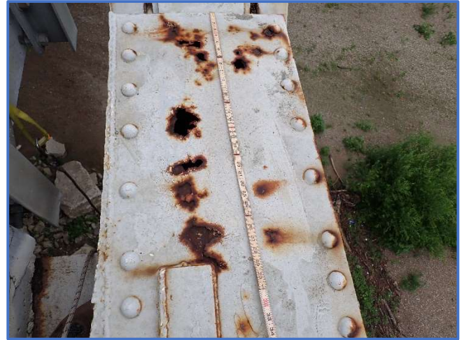
Photo 58 - Corrosion holes with 100% section loss on top cover plate in Span 2, North Truss, at Panel Point 10, looking west
