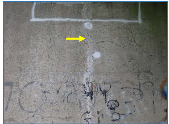
Photo 83 - Crack up to 1/8" wide by full width under Stringer 4 on west face of Pier 4, previously sealed
