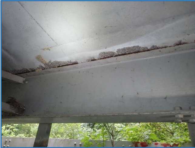
Photo 2 - Typical haunch spall. Shown 15' long by 6" high by 0.5" deep in Span 4, top of Stringer 1, looking north
