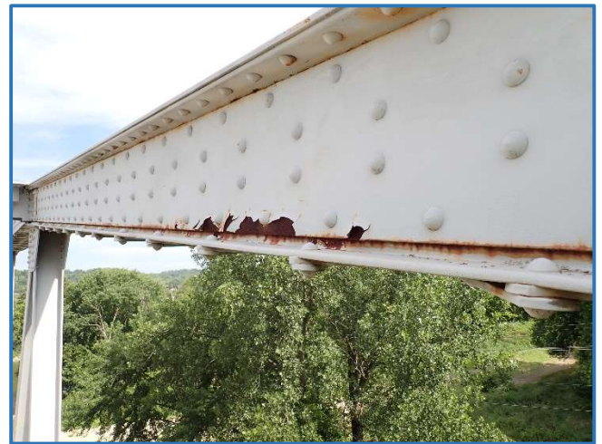
Photo 26 - Reactivated corrosion between the channel and web plate in Span 3, North Truss, member U7U8, looking northwest
