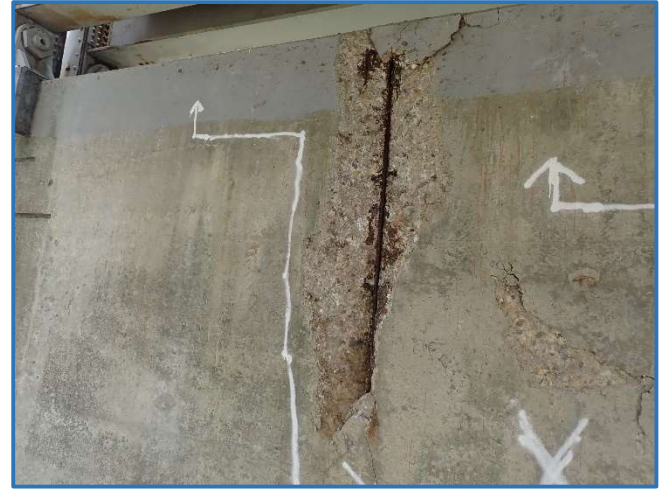
Photo 78 - Spall in west face of Pier 3 under Stringer 2, with exposed rebar with section loss
