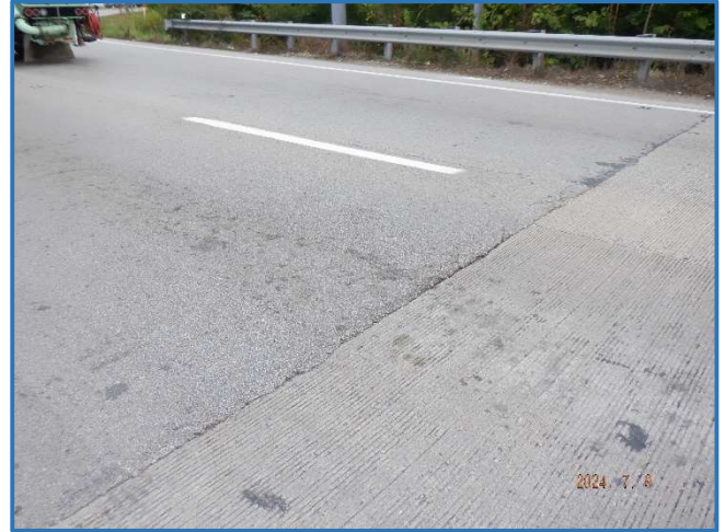
Photo 94 - Map cracking in west approach pavement, looking northwest
