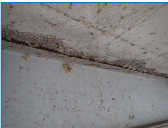
Photo 12 - Typical haunch spalling along outside stringers with surface corrosion along top flange. Shown Span 2, Stringer 1, looking northeast
