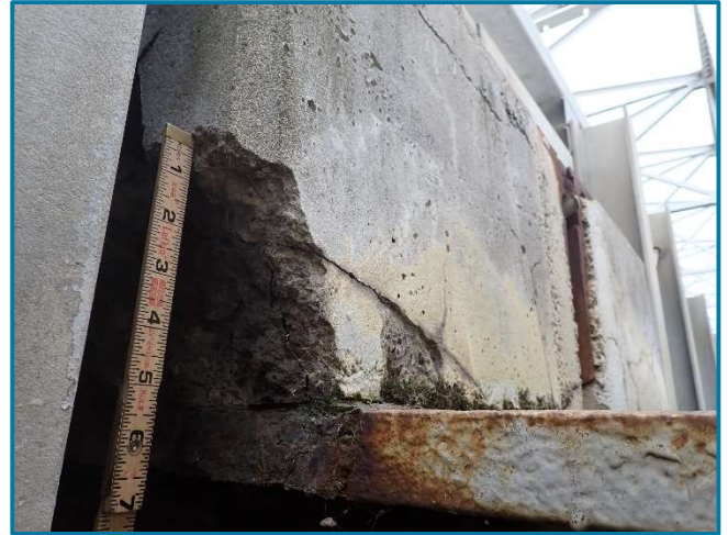
Photo 3 - 6" by 6" by 6" spall on edge of deck on north end, above FBO, in Span 3
