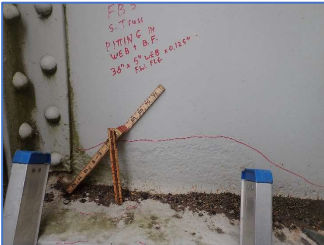
Photo 47 - Pitting along bottom of floorbeam web and top of bottom flange of Floorbeam 5 east face, Span 4, at Stringer 5, looking west
