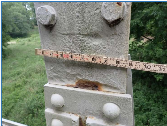
Photo 37 - Pitting with active corrosion and section loss (2" high by 6" wide by 3/8" deep) on vertical just above lower chord connection in Span 3, North Truss, at Panel Point 9, looking west
