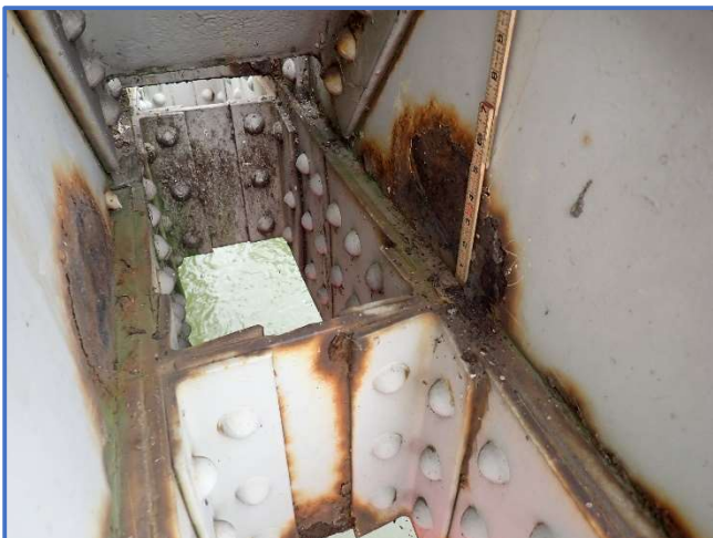
Photo 55 - Laminar corrosion with section loss on interior lower gusset plate. Span 2, North Truss, Panel Point 6, 3" long by 3" wide by 1/8" deep, looking west
