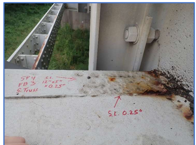
Photo 49 - Pitting with section loss along the top of top flange, at south end of Floorbeam 1, Span 4, looking west
