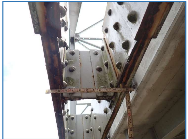
Photo 14 - 1/2" pack rust in lower chord plates in Span 2, North Truss, member L7L8, looking east
