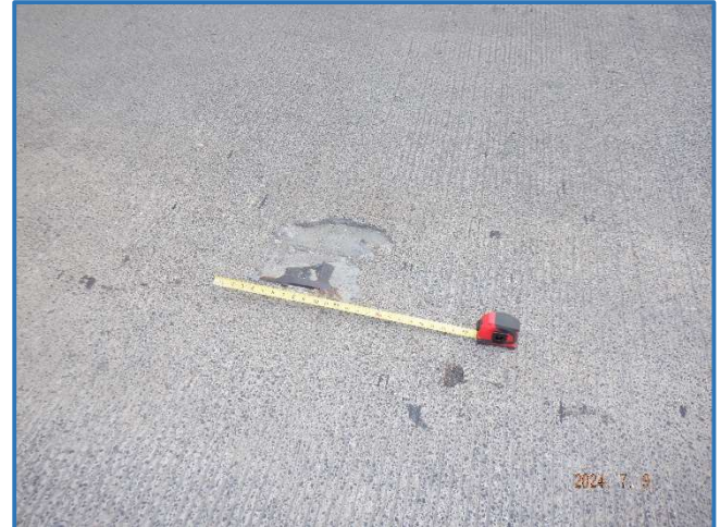
Photo 6 - Spall in Span 1, east side of span
