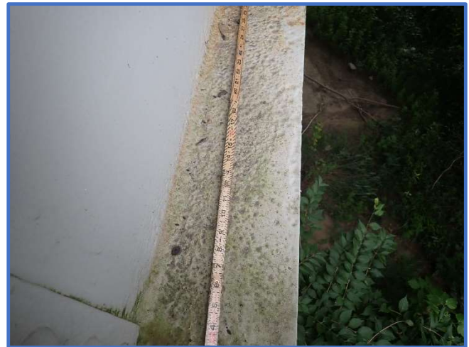
Photo 46 - Typical pitting on top face of bottom flange. Shown is 3.5' long by 1/16" deep pitting on Floorbeam 1, south end, Span 1, looking north
