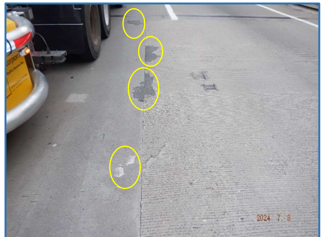
Photo 92 - Spalling in the east approach along center of road, looking west
