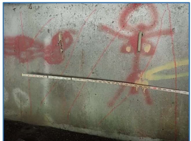
Photo 88 - Delaminated area along backwall of forward abutment
