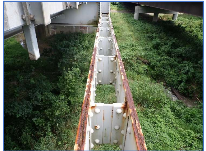
Photo 64 - Typical protective coating condition on lower chord. Shown is Span 3, South Truss, between Panel Points 6 and 7, looking east
