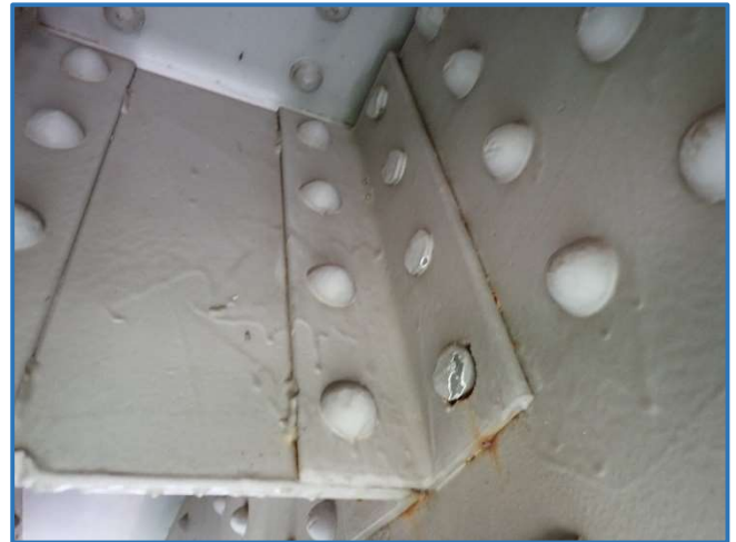
Photo 30 - Typical missing rivet heads on south diaphragm clip angle, Span 3, North Truss, at Panel Point 4, looking southeast
