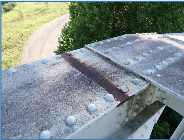
Photo 27 - 6" long by 4" wide paint failure in Span 4, North Truss, member U5U6, looking northeast
