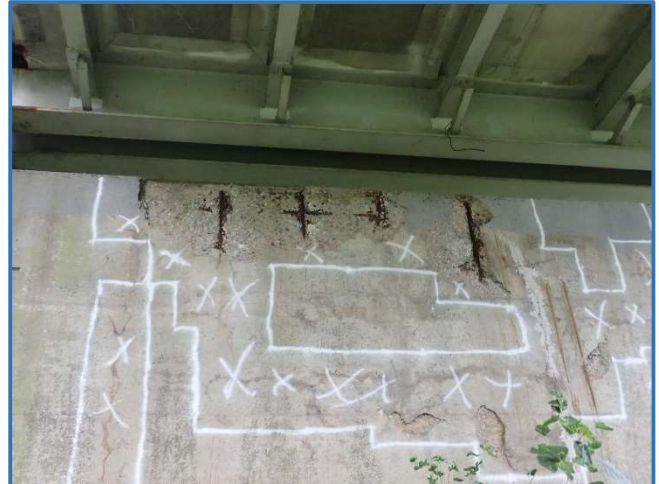
Photo 85 - Spall in Pier 4 west face pier cap, with vertical and transverse rebar exposed
