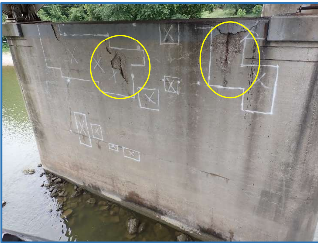
Photo 74 - Large spalls at top of west face of Pier 2
