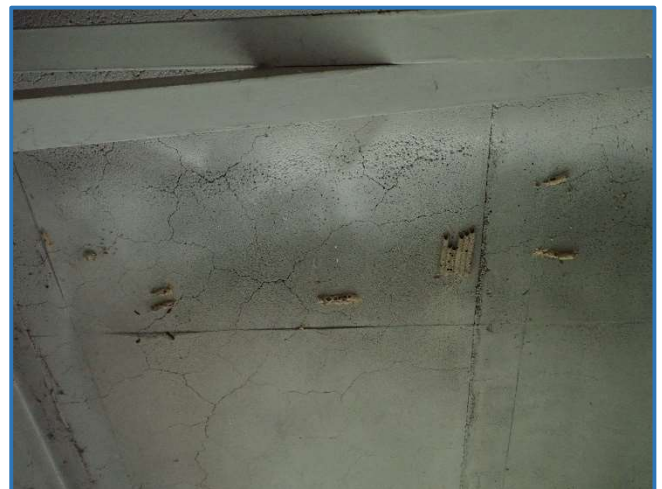
Photo 1 - Typical map cracking in underside deck. Shown Span 4, Bay 3, near Floorbeam 8
