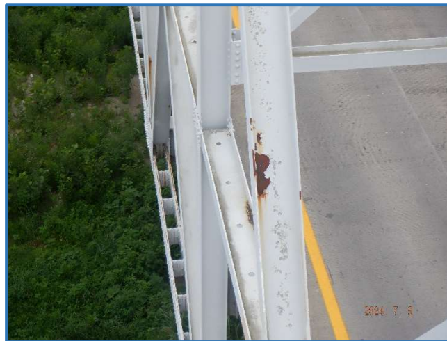
Photo 44 - Paint failure with active corrosion on web of diagonal in Span 3, South Truss, member U5L6, looking west
