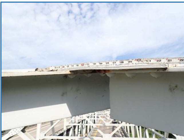
Photo 68 - Bowing in upper lateral bracing connection plate in Span 3, between Panel Points 8 and 9, looking west
