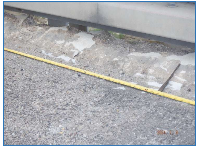
Photo 8 - Spalling of left lane curb in Span 2, between Panel Points 5 and 6
