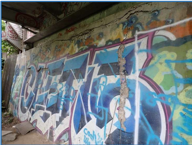
Photo 86 - Rear abutment with cracking and delaminations
