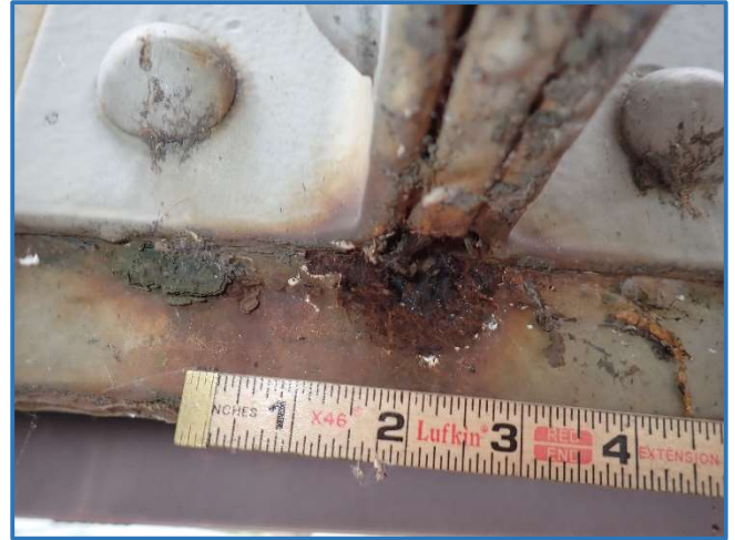
Photo 23 - 2" wide section loss on the web of the lower chord below the vertical connection, Span 1, North Truss, at Panel Point 7, looking south
