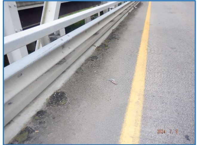
Photo 11 - Typical debris accumulation along edge of bridge deck, shown Span 4, south lane
