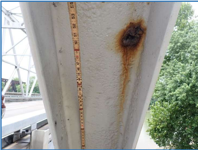
Photo 42 - Pitting on underside of web in Span 2, North Truss, member L8U9, looking west
