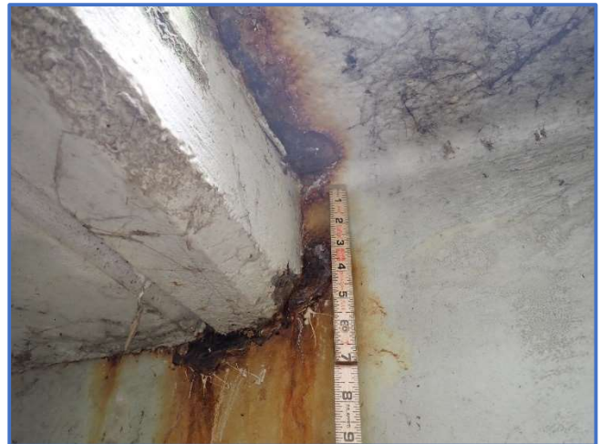
Photo 51 - Corrosion at deck and Floorbeam top flange interface. Shown Span 3, Floorbeam 8, north end, looking west
