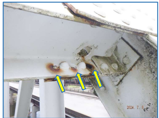
Photo 71 - Misdrilled holes on lower sway brace in portal frame in Span 1, at Panel Point 1, at South Truss connection, looking east
