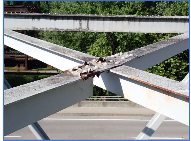
Photo 66 - Typical paint failure of top of upper lateral bracing connection plate with surface corrosion. Shown in Span 4, between Panel Points 3 and 4, looking south
