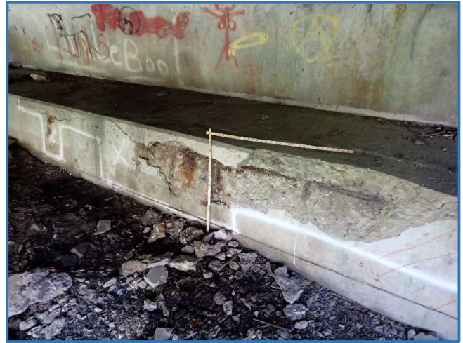
Photo 89 - Delamination and spalling with exposed rebar along bearing seat of forward abutment, looking southeast
