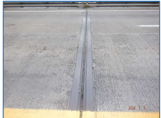
Photo 7 - Typical expansion joint with debris and surface corrosion. Shown is Pier 2 joint, looking north
