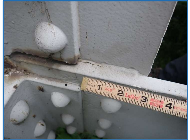
Photo 19 - Tack weld between lower chord plate and gusset plate, Span 1, South Truss, Panel Point 1, looking north
