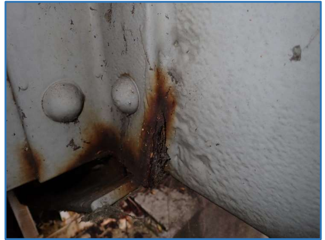
Photo 21 - Area of 2" wide by 4" high x 3/16" deep pitting on the south face of north web plate in Span 1, North Truss, between Panel Point 0 and 1, looking west
