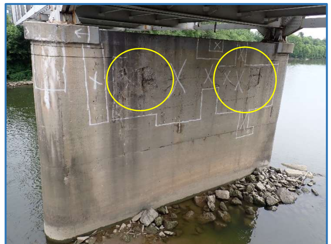
Photo 76 - Large spalls at top of east face of Pier 2
