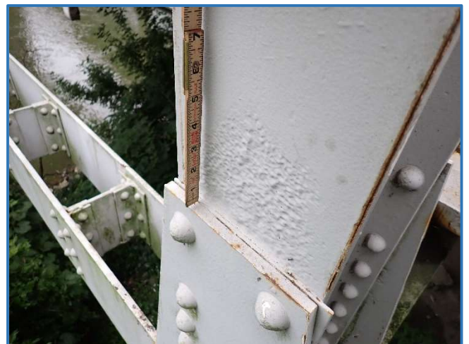
Photo 38 - Painted over pitting up to 3/16" deep on vertical just above lower chord connection, Span 1, North Truss, at Panel Point 1, looking northwest
