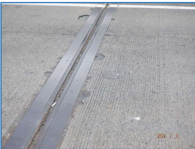
Photo 4 - Spalling along Pier 2 joint
