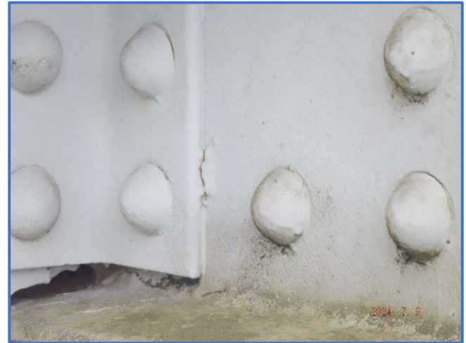
Photo 33 - Crack in tack weld between upper chord and sway bracing connection plate in Span 4, South Truss, at Panel Point 4, looking southeast
