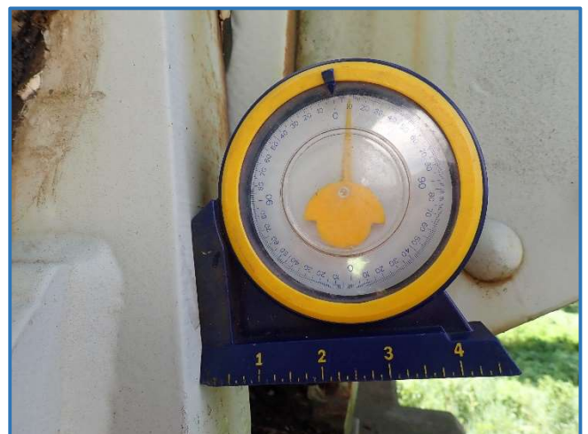
Photo 60 - 9-degree tilt of bearing in Span 3, north bearing on Pier 4, looking south
