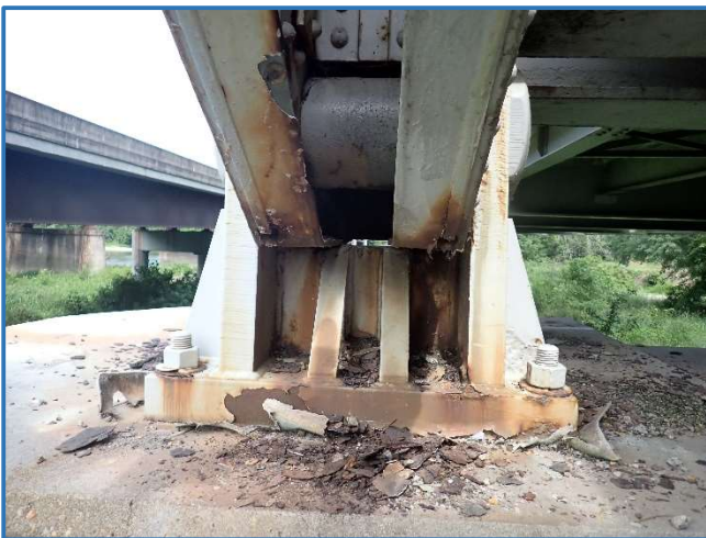
Photo 59 - Typical corrosion and section loss on bearings. Shown is Span 3, movable bearing on Pier 4, looking east
