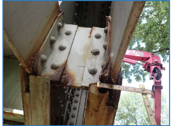
Photo 17 - Bowing in lower chord northeast diaphragm angle due to pack rust, 1 1/2" over 4", Span 4, North Truss, member L0L1
