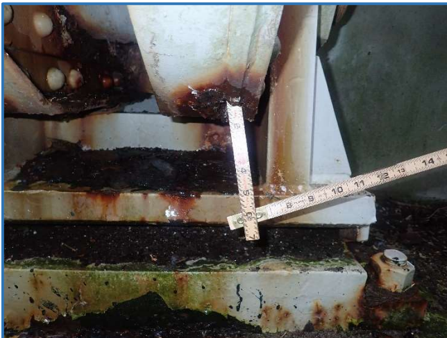
Photo 22 - Up to 100% section loss on the lower chord stiffener, Span 4, North Truss, at L8, looking east
