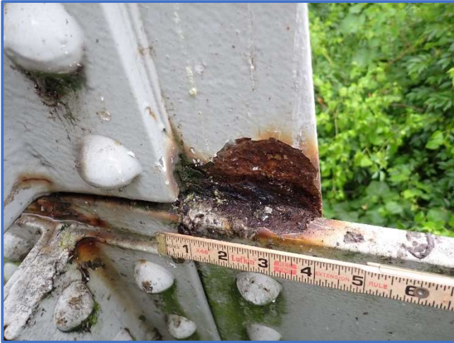
Photo 57 - Section loss on east edge of lower gusset plate at top of lower chord, Span 1, North Truss, at Panel Point 1, looking north
