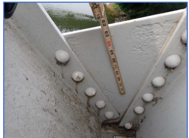
Photo 56 - Typical coated pitting on interior gusset plate. Shown Span 1, South Truss, at Panel Point 4, looking south
