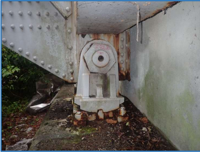
Photo 61 - 5-degree tilt of north bearing at forward abutments, looking north
