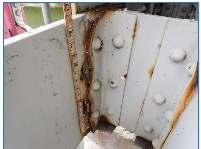
Photo 16 - 3/4" pack rust between lower chord and diaphragm, Span 2, South Truss, member L0L1
