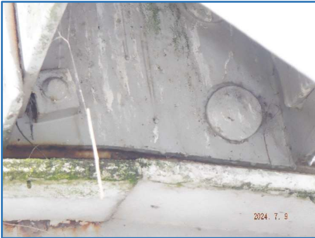
Photo 32 - Bolt with square nut and flattened rivet head on upper chord stiffener plate, Span 2, South Truss, at Panel Point 3, looking south
