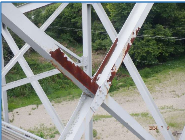
Photo 72 - Surface corrosion on diagonal sway braces in Span 3, at Panel Point 3, looking west
