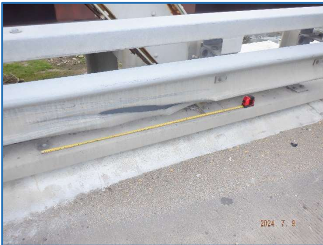
Photo 9 - Impact damage to metal railing, showing Span 3, south railing, between Panel Points 0 and 1
