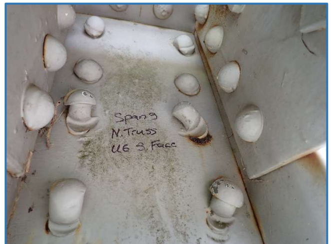
Photo 31 – Improperly installed rivets in stiffener plate, Span 3, North Truss, at Panel Point 6, looking north
