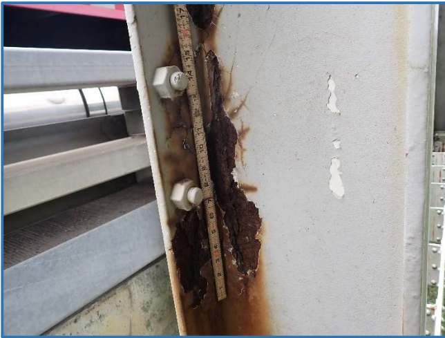
Photo 39 - Laminar corrosion on flange and web of vertical member in Span 3, North Truss, at Panel Point 9, looking west
