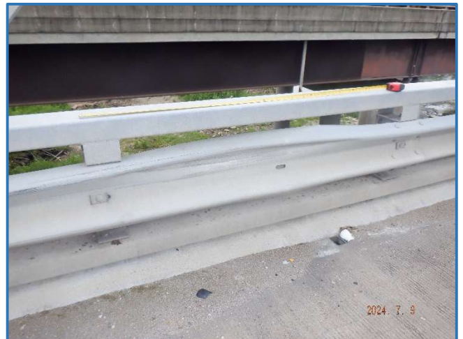
Photo 10 - Impact damage to metal railing, showing Span 3, south railing, between Panel Points 1 and 2
