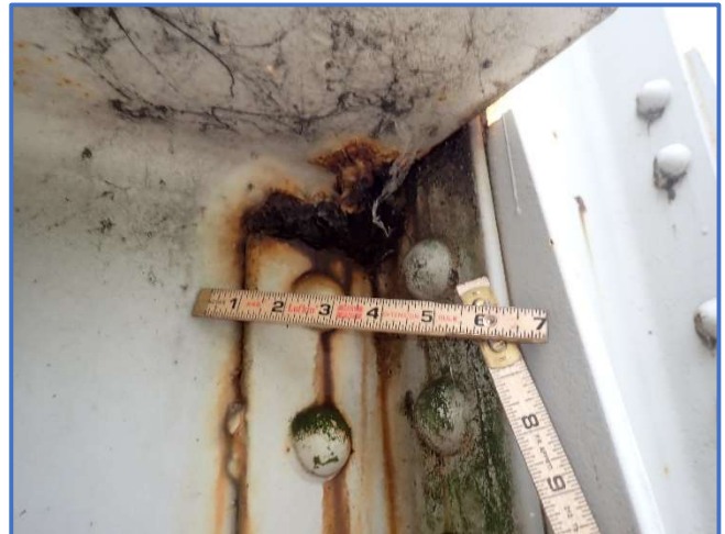
Photo 54 – Corrosion along top flange and clip angle in Span 2, Floorbeam 9 west face, north end, looking west. Note tack weld at clip angle to floorbeam web connection.
