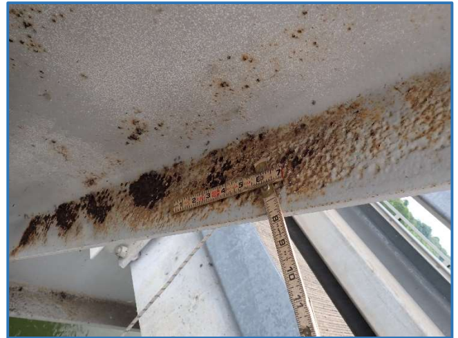
Photo 43 - Pitting on interior of flange in Span 1, South Truss, member L5U6, looking northwest
