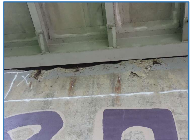
Photo 84 - Spall in top of Pier 3 east face between Stringers 2 and 4, with exposed rebar
