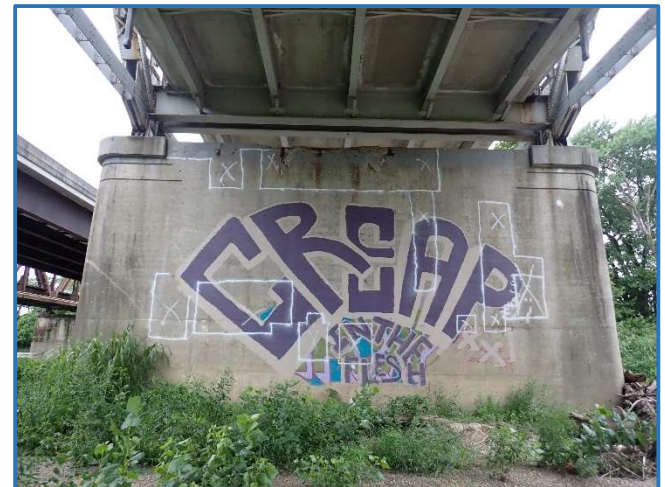
Photo 79 - Widespread delaminated areas and spalls on east face of Pier 3
