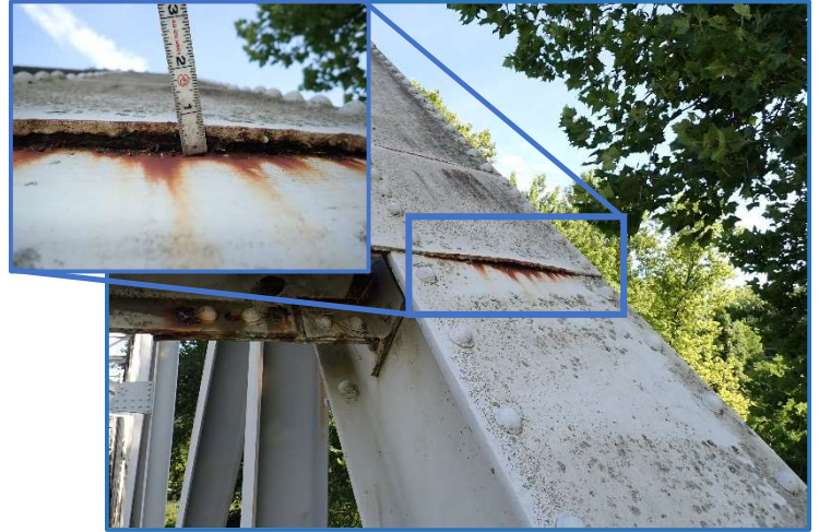
Photo 36 - 1/2" pack rust between portal bracing connection plate and edge post in Span 4, North Truss, on U7L8, looking west
