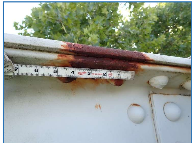
Photo 28 - 6" long by 4" wide paint failure in Span 4, North Truss, member U6U7, looking north
