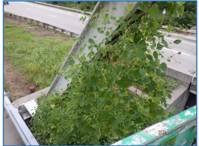
Photo 96 - Vegetation growth along underside of end post in Span 4, South Truss, between Panel Points 7 and 8, looking northeast
