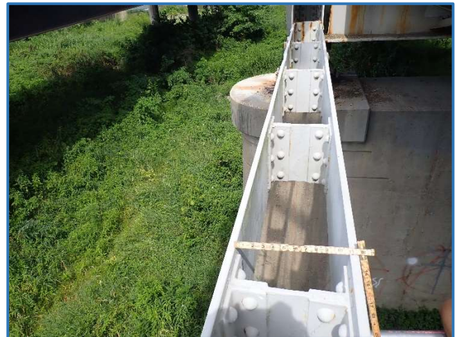
Photo 18 - Inconsistent diaphragm dimensions; Member L0L1, South Truss, Span 4 shown
