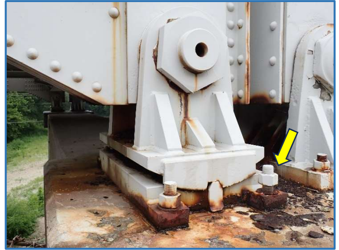
Photo 62 - Backed off nut on southeast anchor bolt on south bearing in Span 2, at Pier 3, looking north
