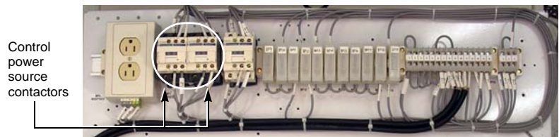
Figure 15: Control Power Source Contactor
