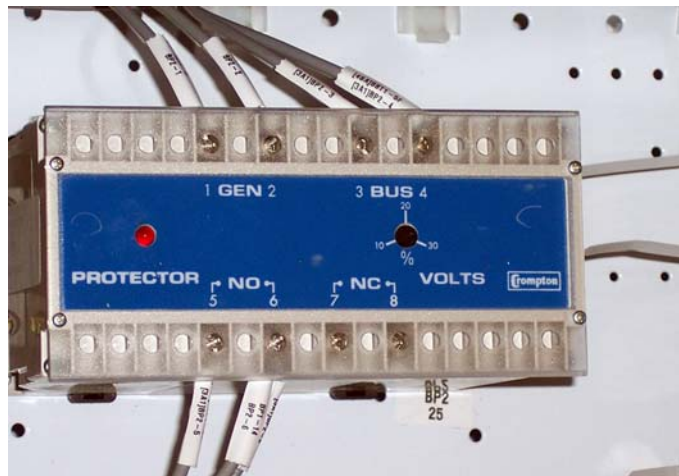
Figure 13: Sync-Check Relay Assembly
