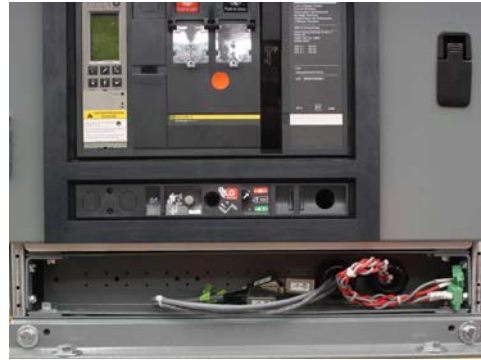
Figure 33: Example of Communication Cables Temporarily Stored in Wireway for Shipment
