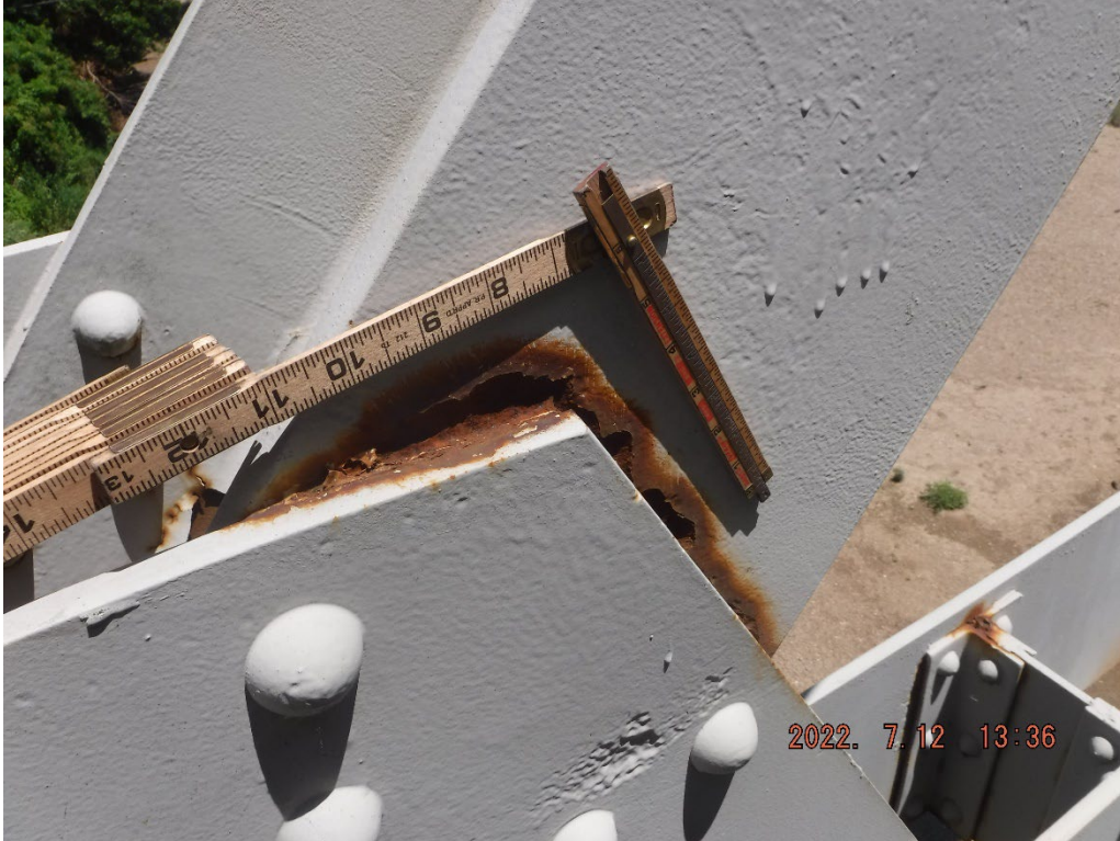
Photo 38: Active pitting up to 3/16" deep on L8U9, Span 2, North Truss
