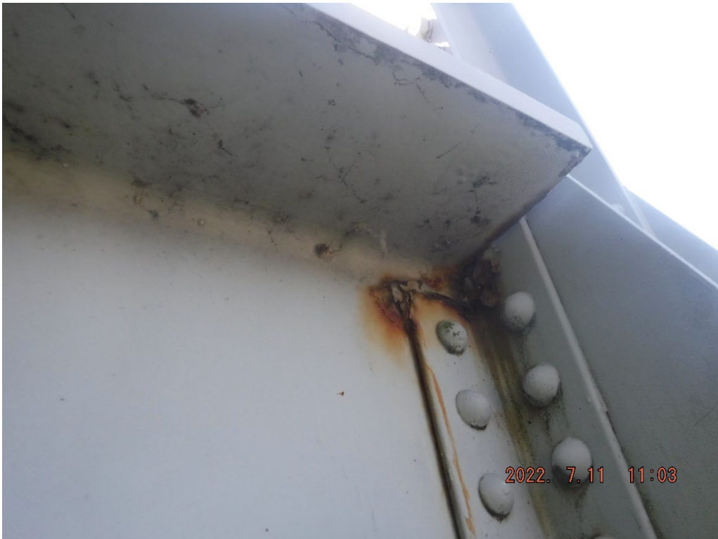
Photo 46: Laminating corrosion and pack rust at FB7 connection to gusset plate, Span 3, South end
