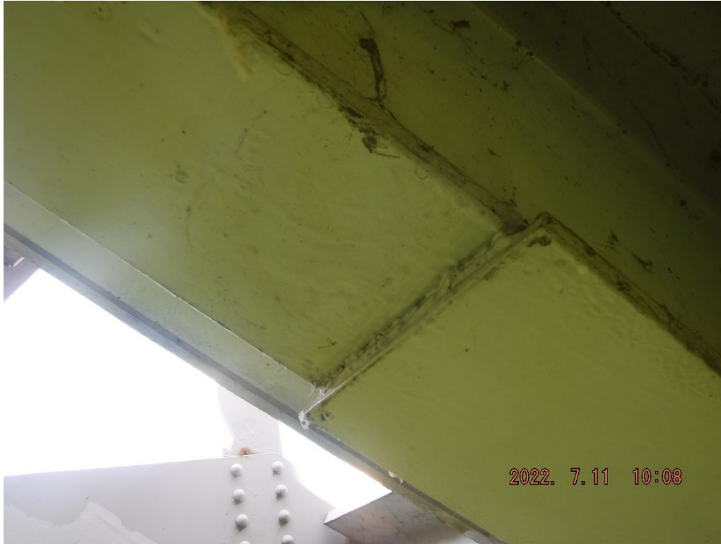
Photo 14: Typical poor quality weld between stringer and coverplate (S1 at FB6 in Span 3 shown)
