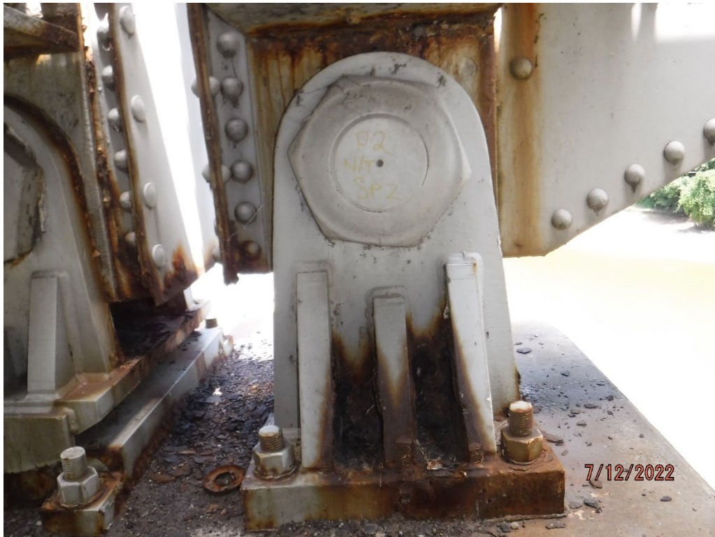
Photo 58: Active corrosion with minor section loss on North bearing, Span 2, Pier 2
