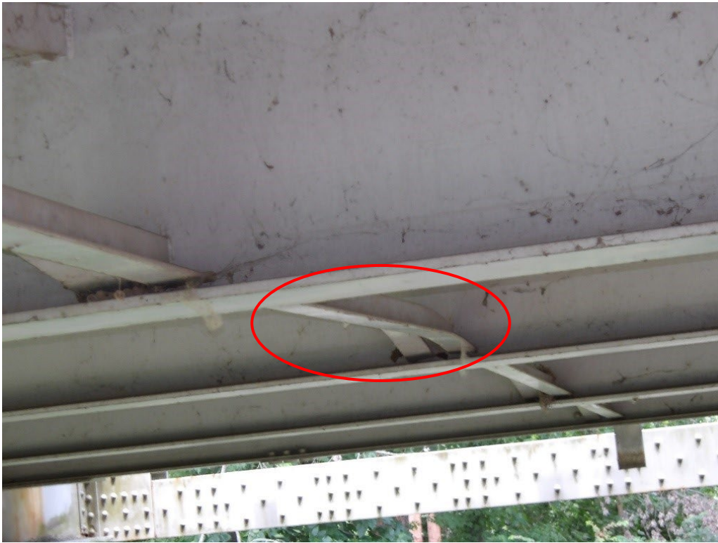
Photo 64: Bent stringer cross frame between FB4 and FB5 in Span 4
