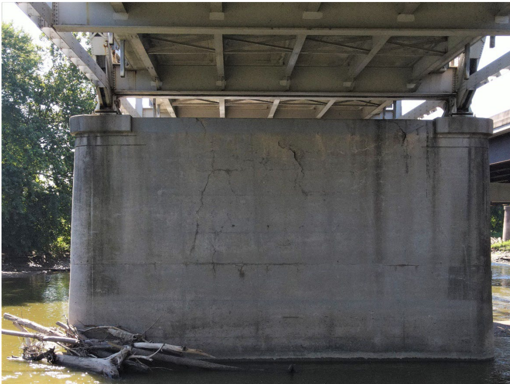
Photo 68: Cracks and delaminations on west face of Pier 2
