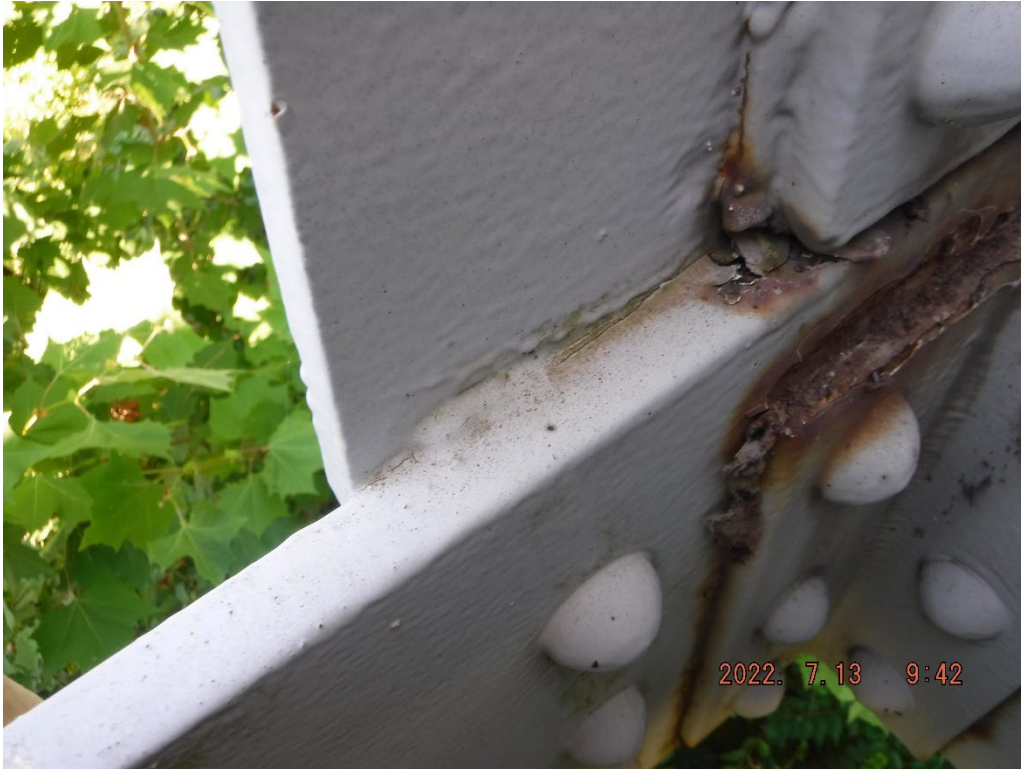
Photo 25: Tack weld between lower chord and gusset plate at L1, Span 1, South Truss
