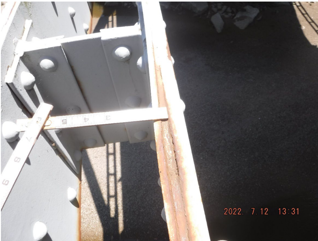
Photo 16: Active pack rust up to 1/2" thick on L7L8, Span 2, North Truss
