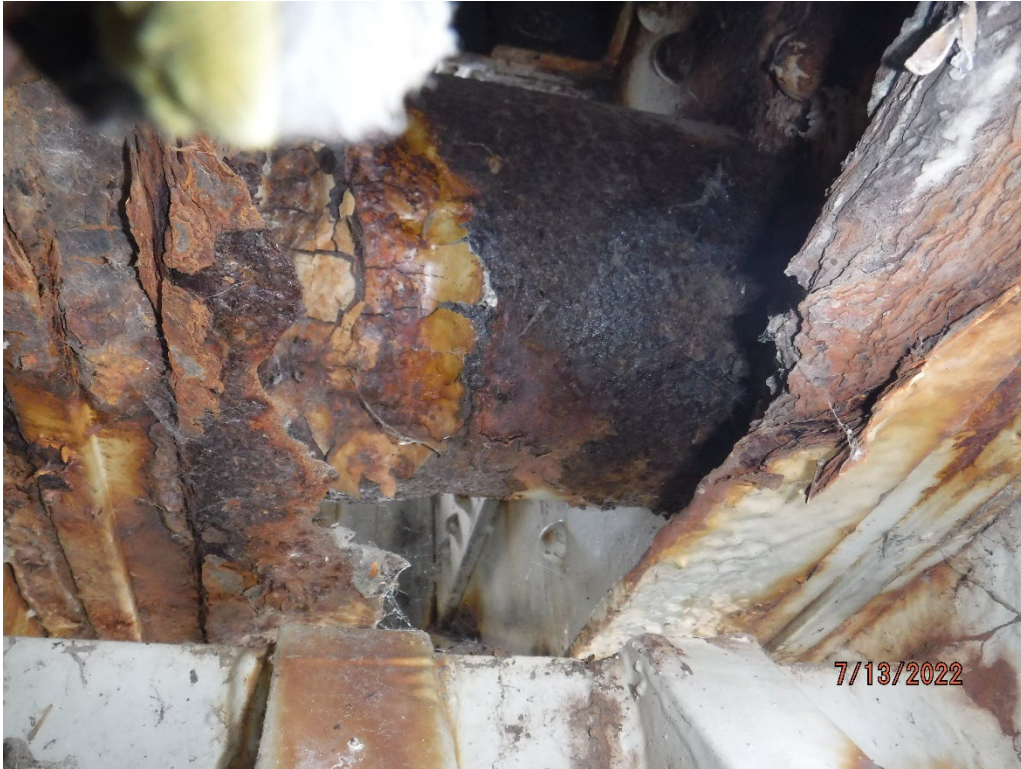
Photo 54: Laminating corrosion on the south bearing pin at Span 3, Pier 3
