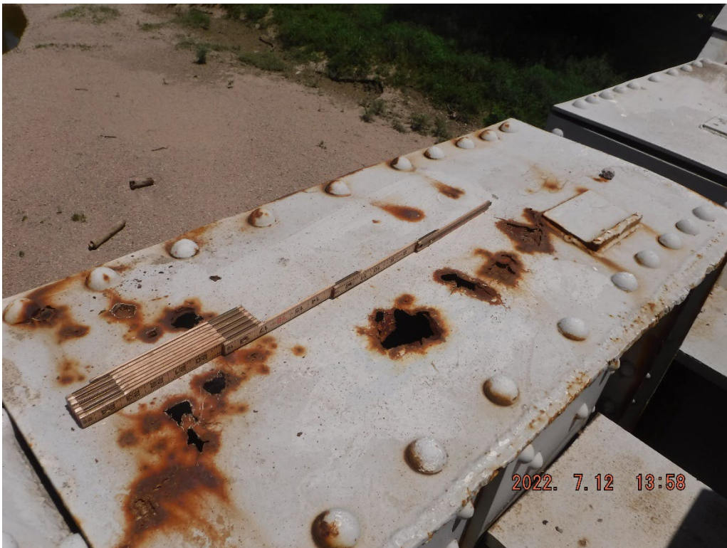
Photo 55: Corrosion holes in top cover plate of L10, Span 2, North Truss
