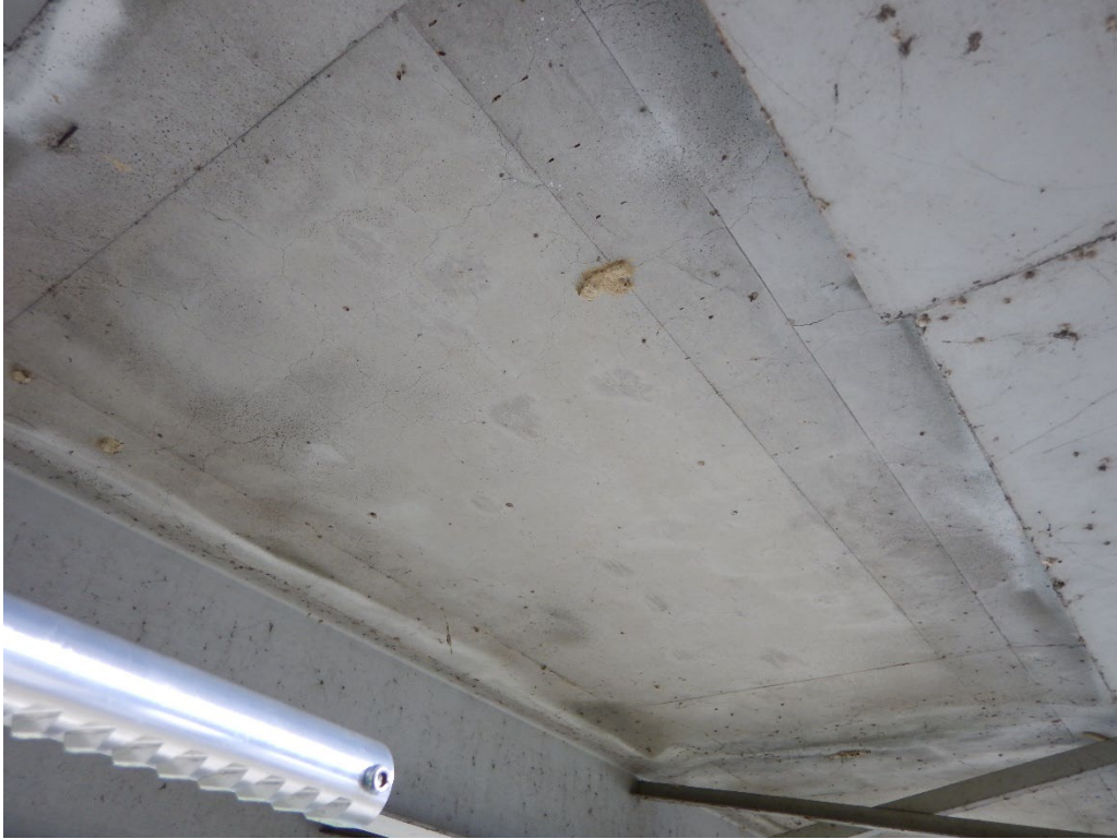
Photo 2: Typical map cracking throughout the deck underside (Span 1 shown)
