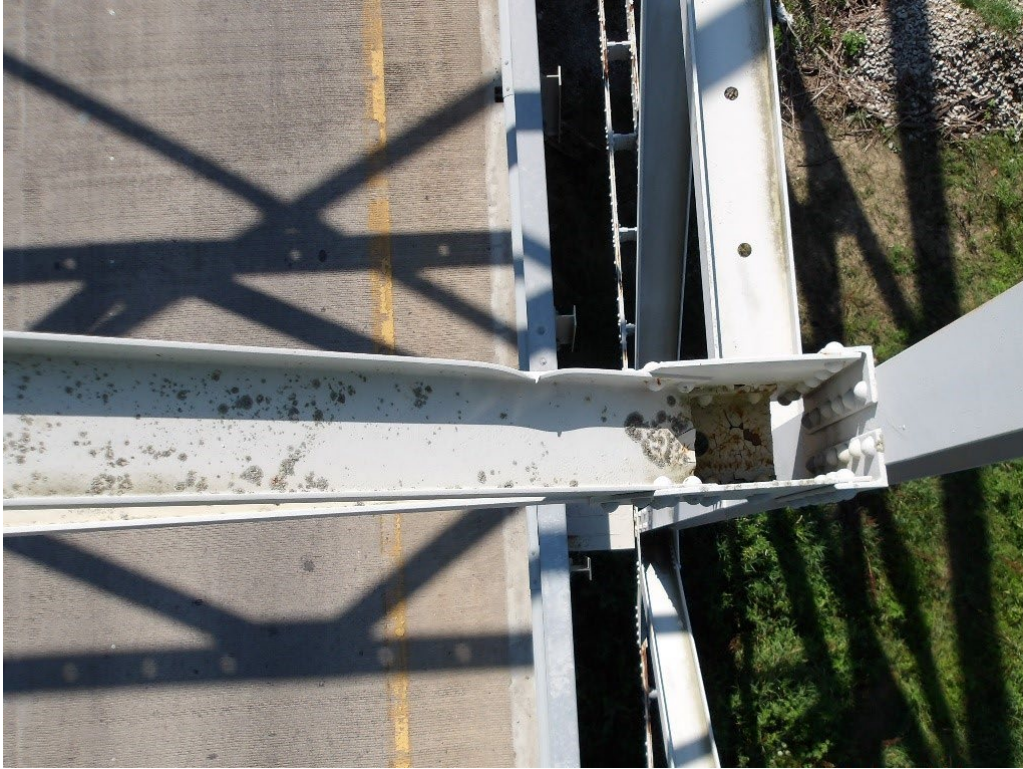
Photo 66: Impact damage of the sway bracing member in Span 4 below U3
