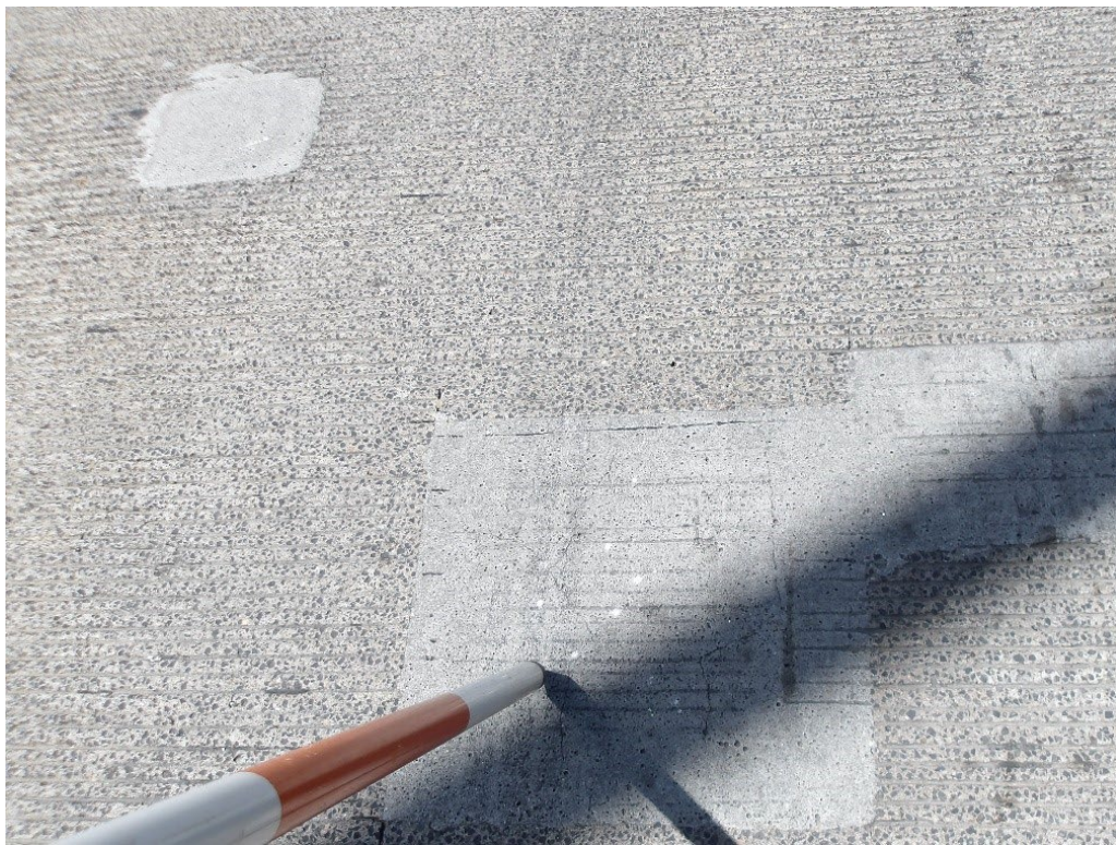
Photo 4: Deck patches with hairline cracks in Span 2
