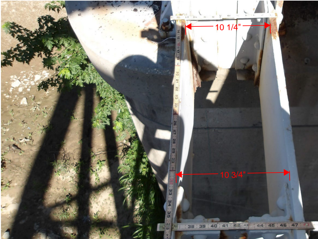
Photo 23: Inconsistent diaphragm dimensions causing bowing in LOL1 at L0, Span 3, South Truss
