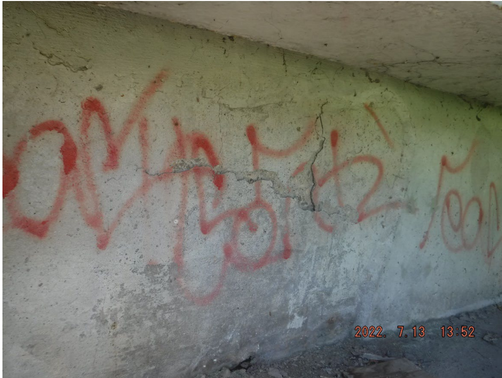
Photo 79: Cracks and delaminations in Rear Abutment backwall
