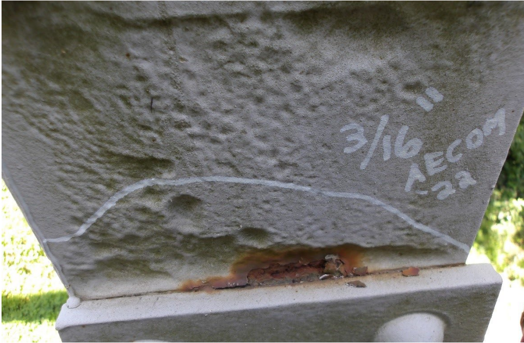
Photo 33: Section loss in U9L9, Span 3, North Truss
