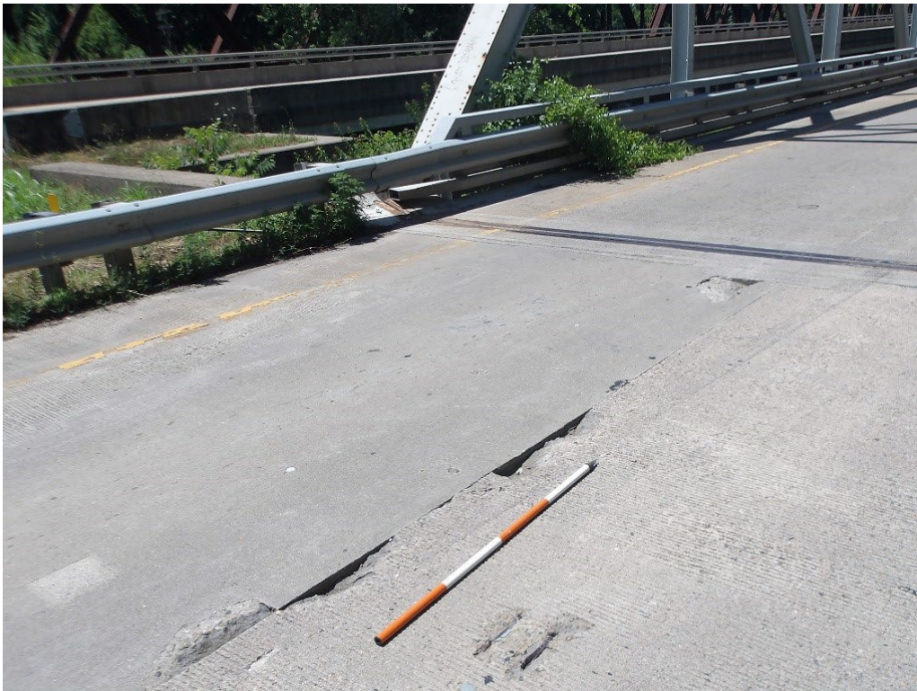
Photo 82: Spalls in Forward Approach Slab
