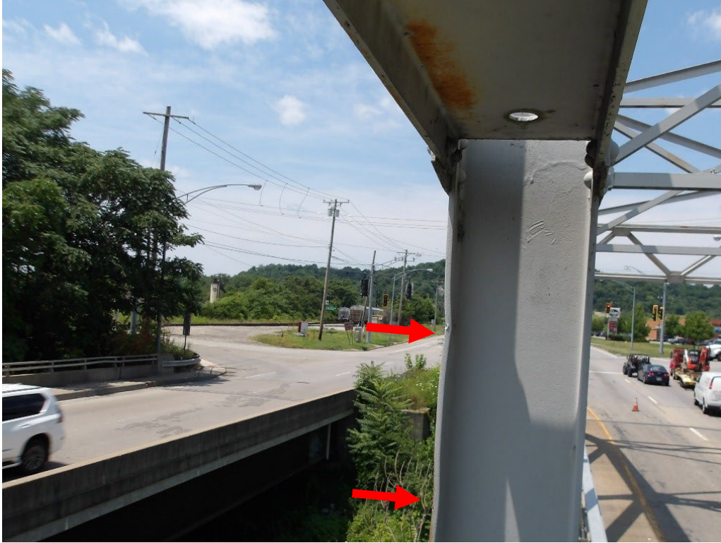
Photo 37: Deformations of L4U4, Span 1, South Truss
