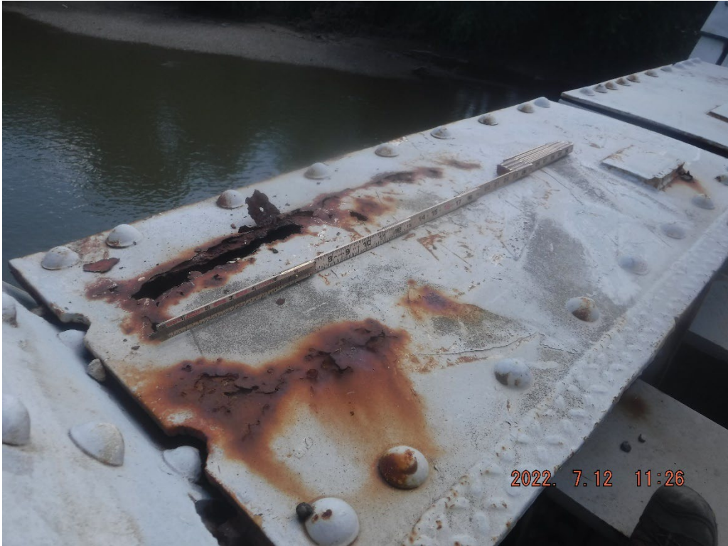
Photo 56: Corrosion holes in top cover plate of L8, Span1, North Truss
