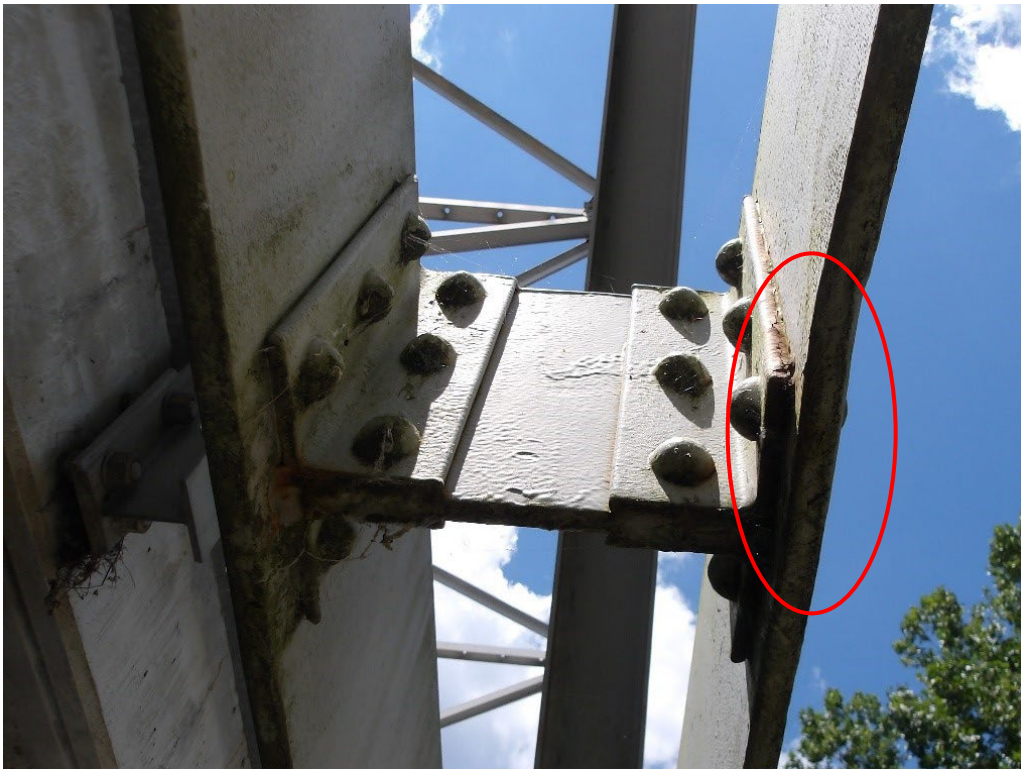
Photo 24: Bow on outboard plate of L6L7, Span 4, North Truss
