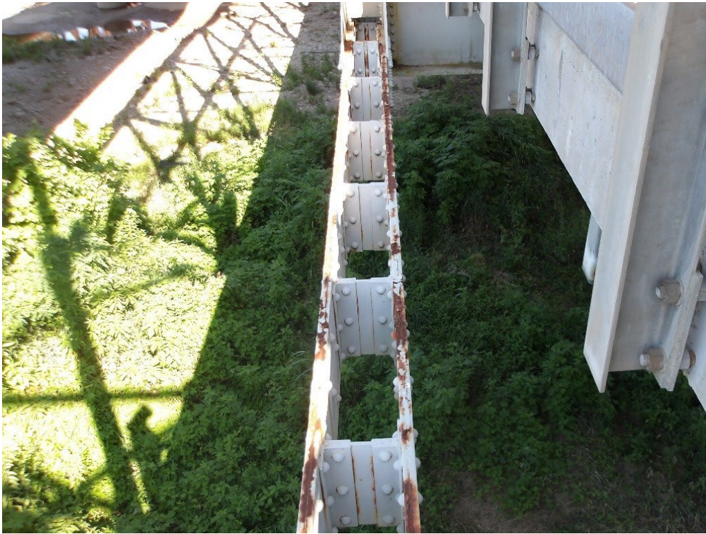
Photo 62: Typical lower paint condition (L6L7 at Span 3, South Truss shown)
