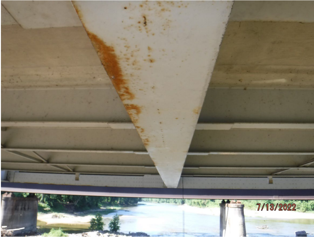
Photo 63: Typical floorbeam freckling corrosion (FB7, Span 2 looking South shown)
