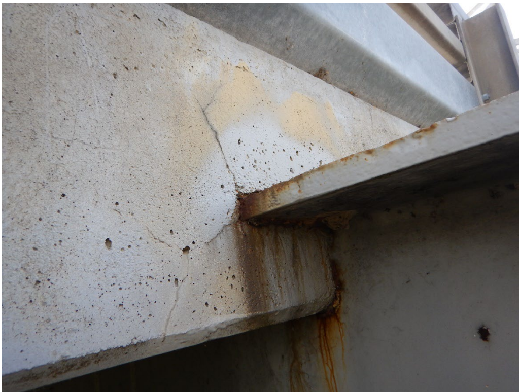
Photo 3: Hairline radial cracking in deck edge at Floorbeam 2 in Span1
