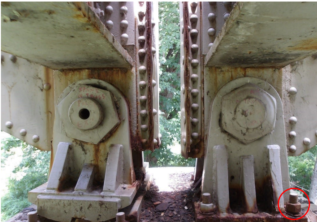
Photo 60: Loose anchor nut and laminating corrosion at North bearings, Pier 4
