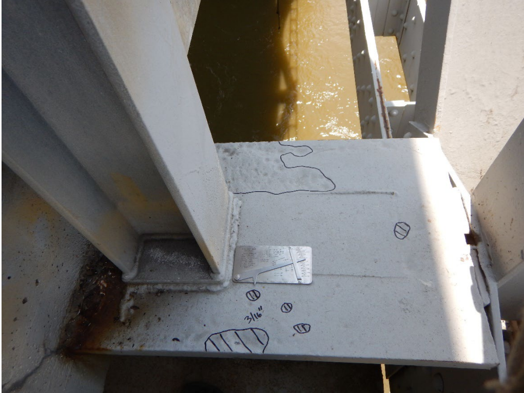
Photo 43: Pitting up to 3/16" deep in top flange of FB 4, Span 1, South end
