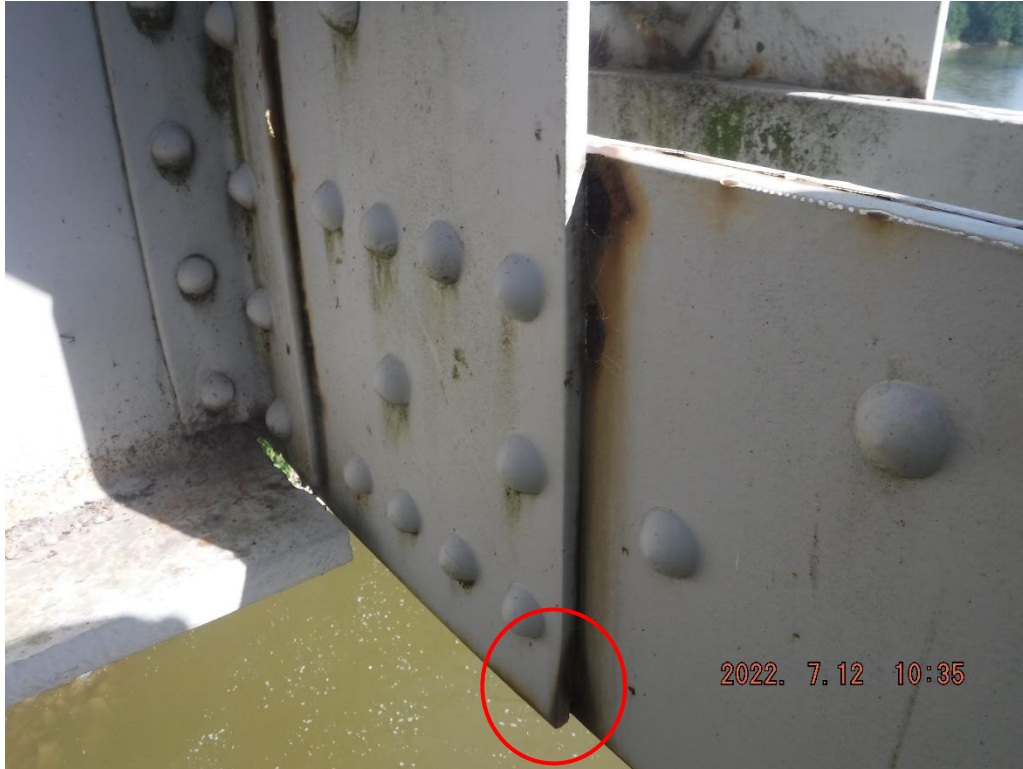
Photo 48: Pack rust deforming L4 gusset plate up to 1/4" in Span 1, North Truss
