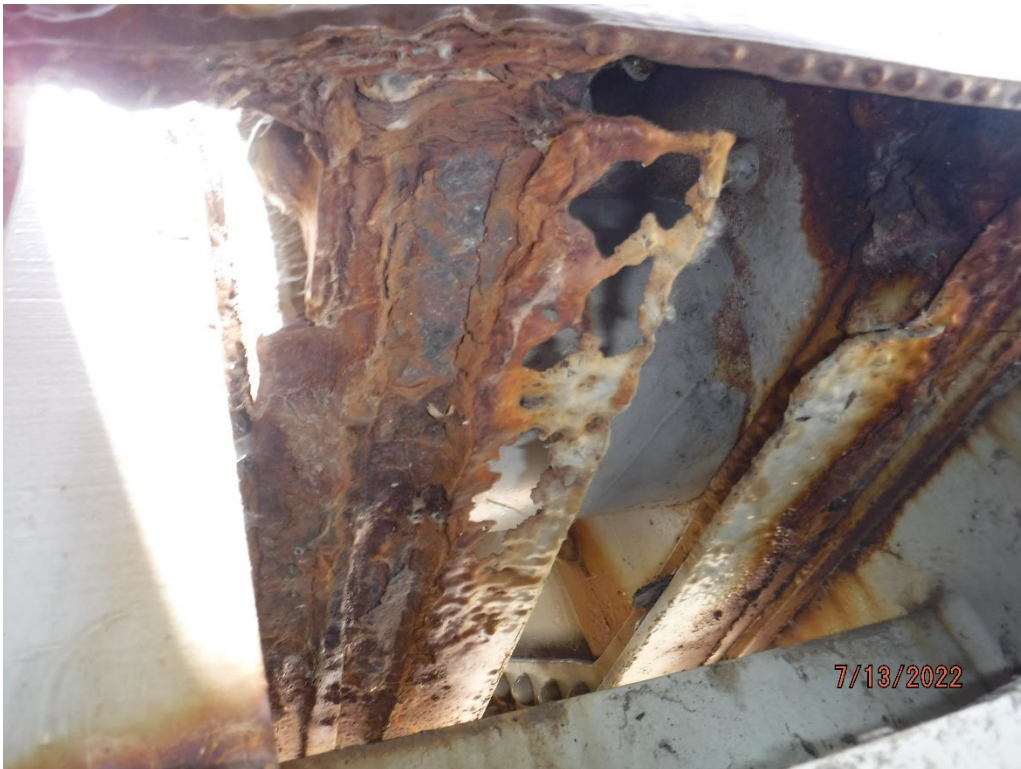
Photo 53: Corrosion holes in L0 gusset plate stiffening angles behind Pier 3 bearing, Span 3, North Truss
