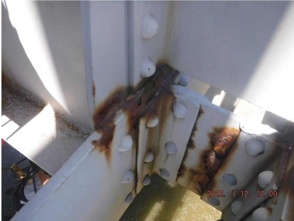
Photo 21: Laminating corrosion on L1L2, Span 2, North Truss
