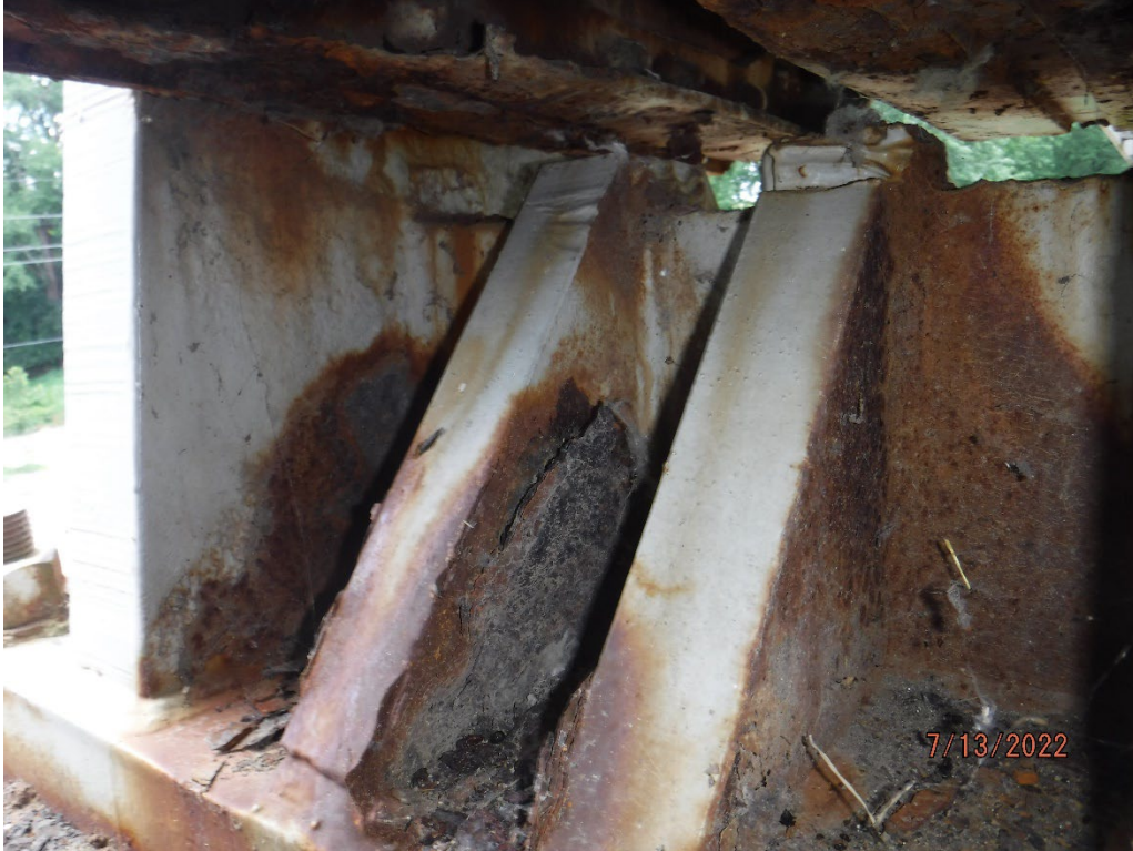
Photo 59: Laminating corrosion with section loss at North bearing, Span 3, Pier 3
