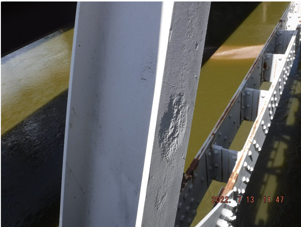
Photo 39: Painted over pitting on U3L4, Span 2, South Truss
