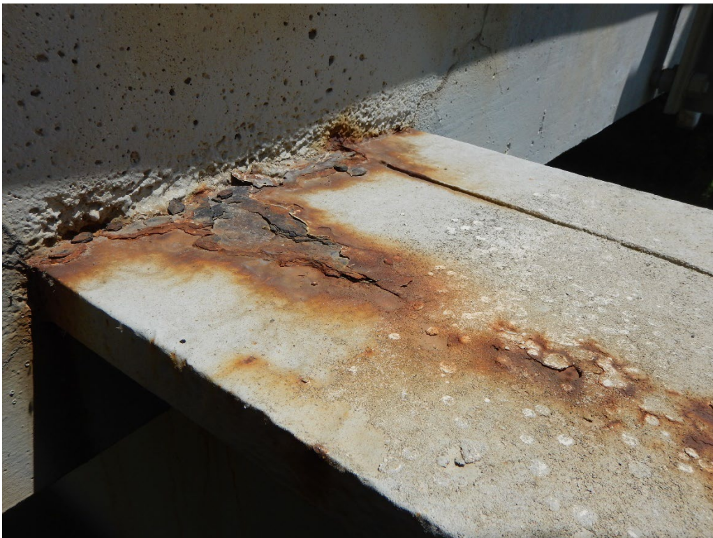
Photo 44: Laminating corrosion on top flange of FB 5, Span 3, South end
