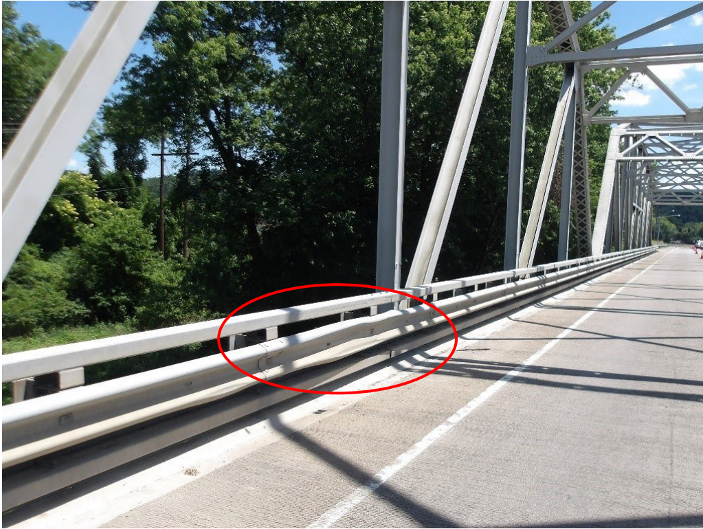
Photo 10: Impact damage to north railing in Span 3
