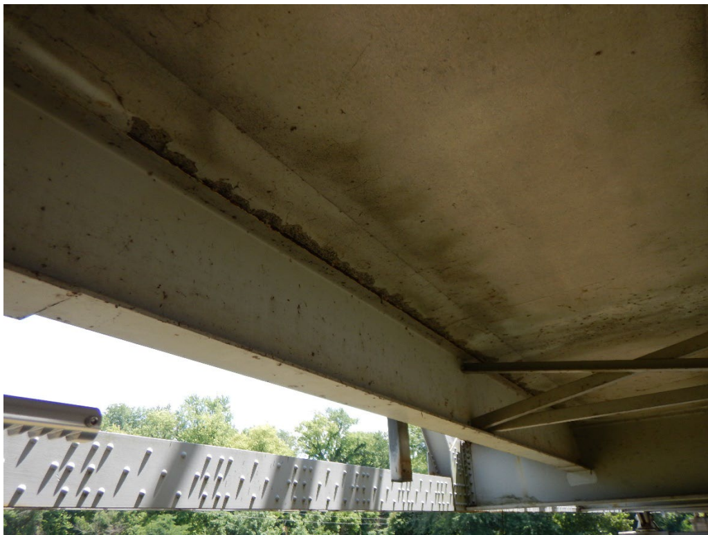
Photo 13: Typical stringer surface corrosion at haunch spalls
