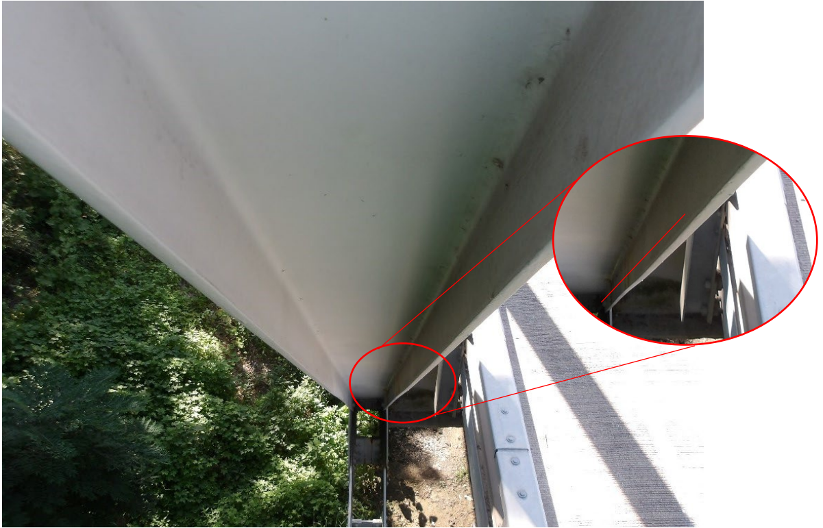
Photo 40: Bowing of inboard flange of U1L2, Span 4, North Truss
