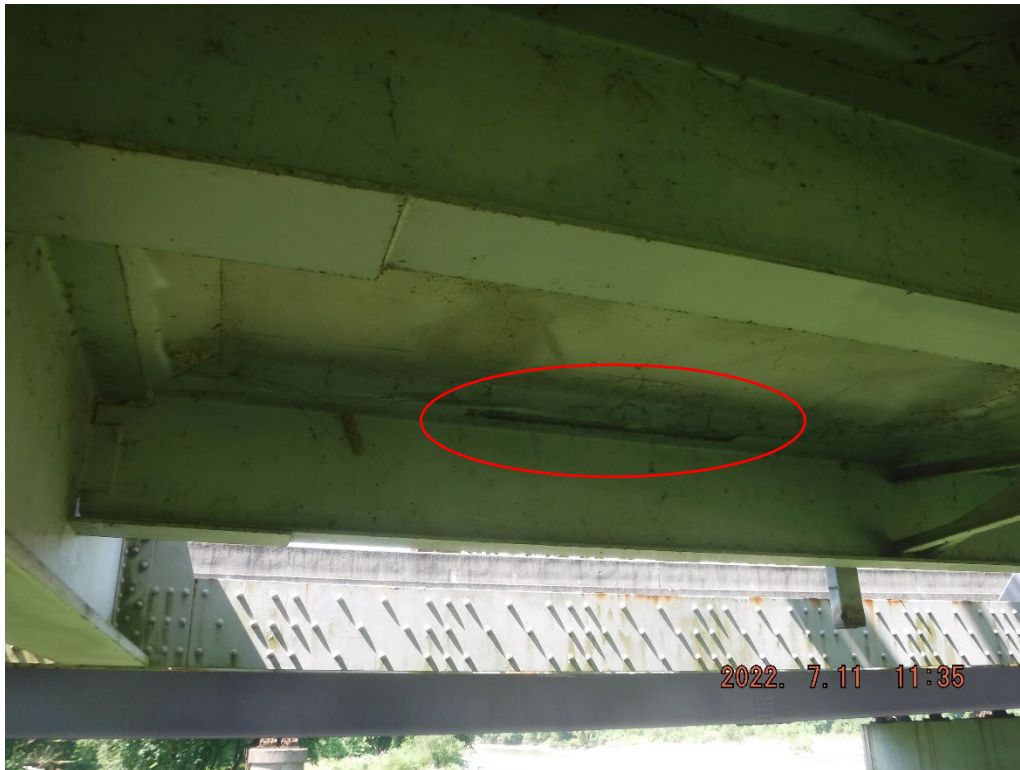
Photo 1: Typical haunch spall (Bay 5 in Span 3 shown)
