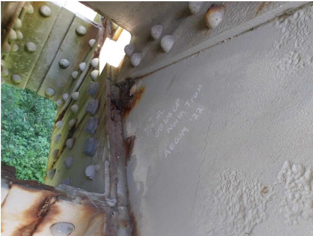
Photo 51: Pitting in L8, Span 3, North Truss
