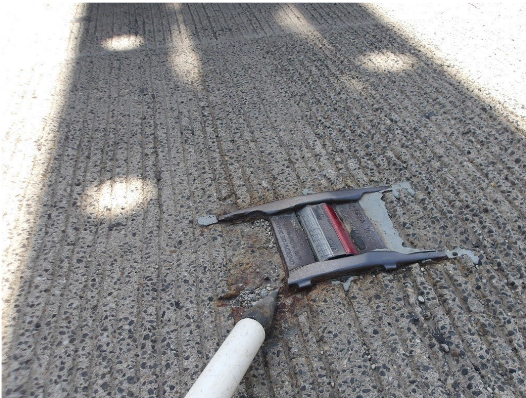
Photo 6: Broken RPM with sharp metal edge in Span 4
