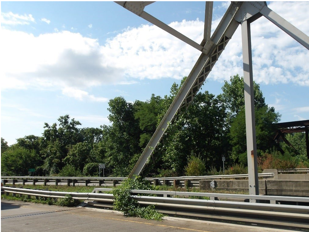
Photo 31: Vegetation grown on end post LOU1, Span 4, South Truss
