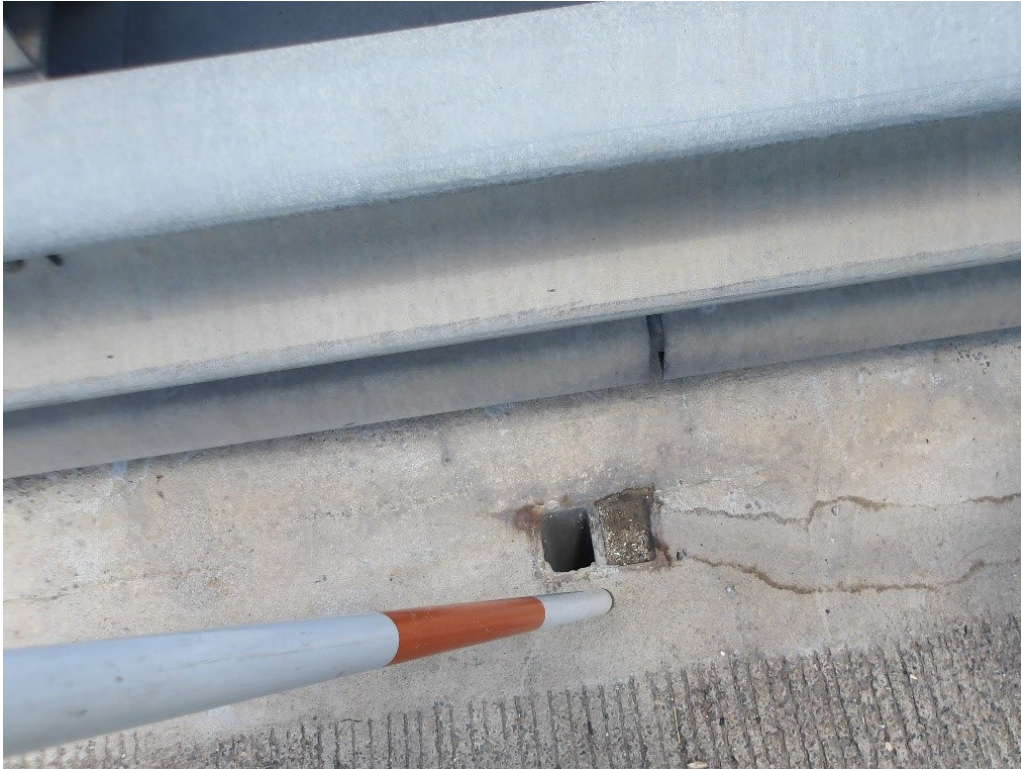
Photo 12: Partially clogged drain
