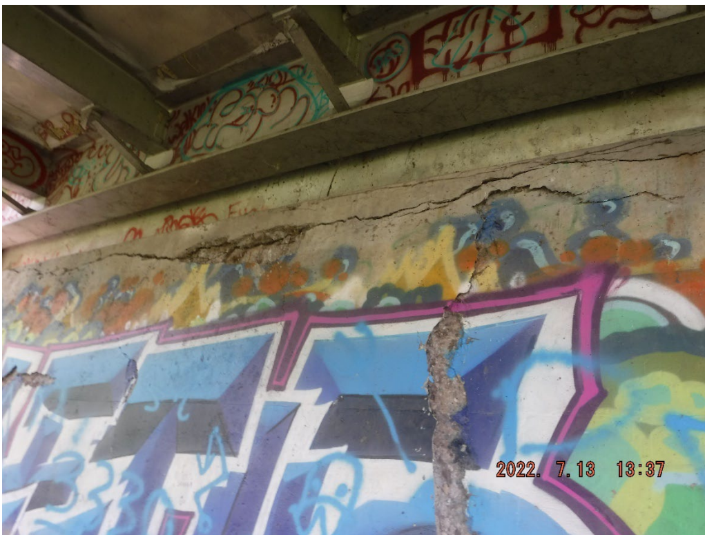
Photo 73: Spalls, cracks and delaminations on Rear Abutment
