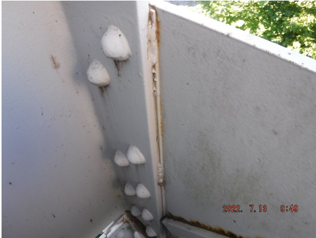
Photo 35: Undercut tack welds between the vertical and fill plate, L2U2, Span 1, South Truss
