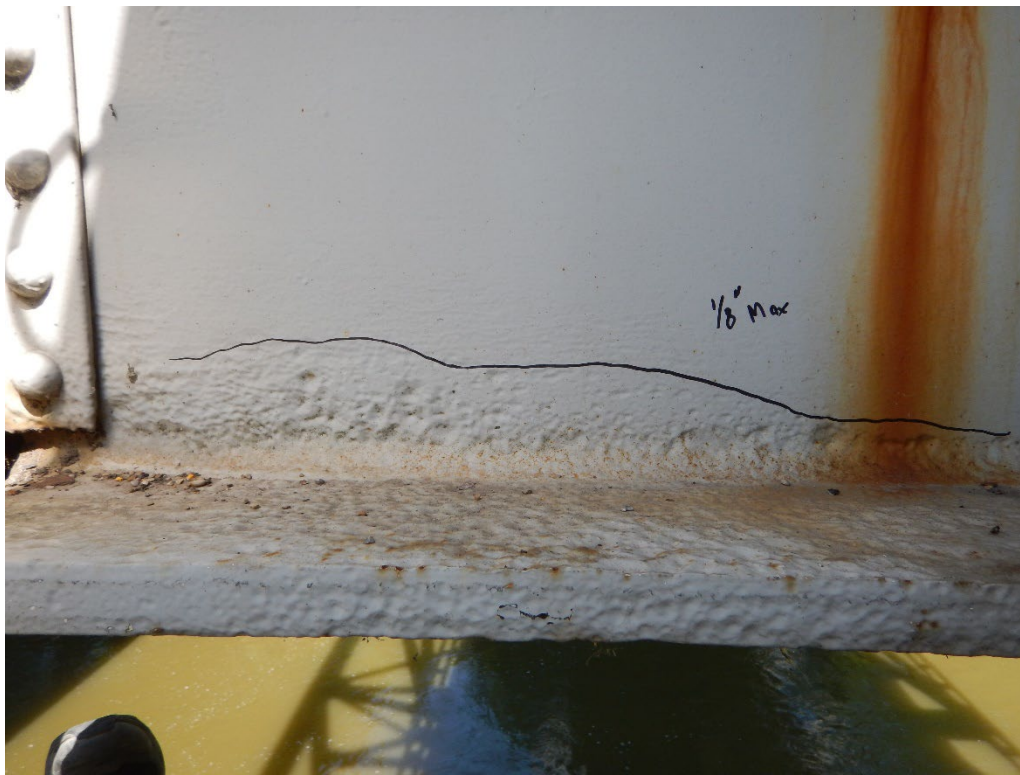
Photo 42: Pitting up to 1/8" deep in FB6, Span 1
