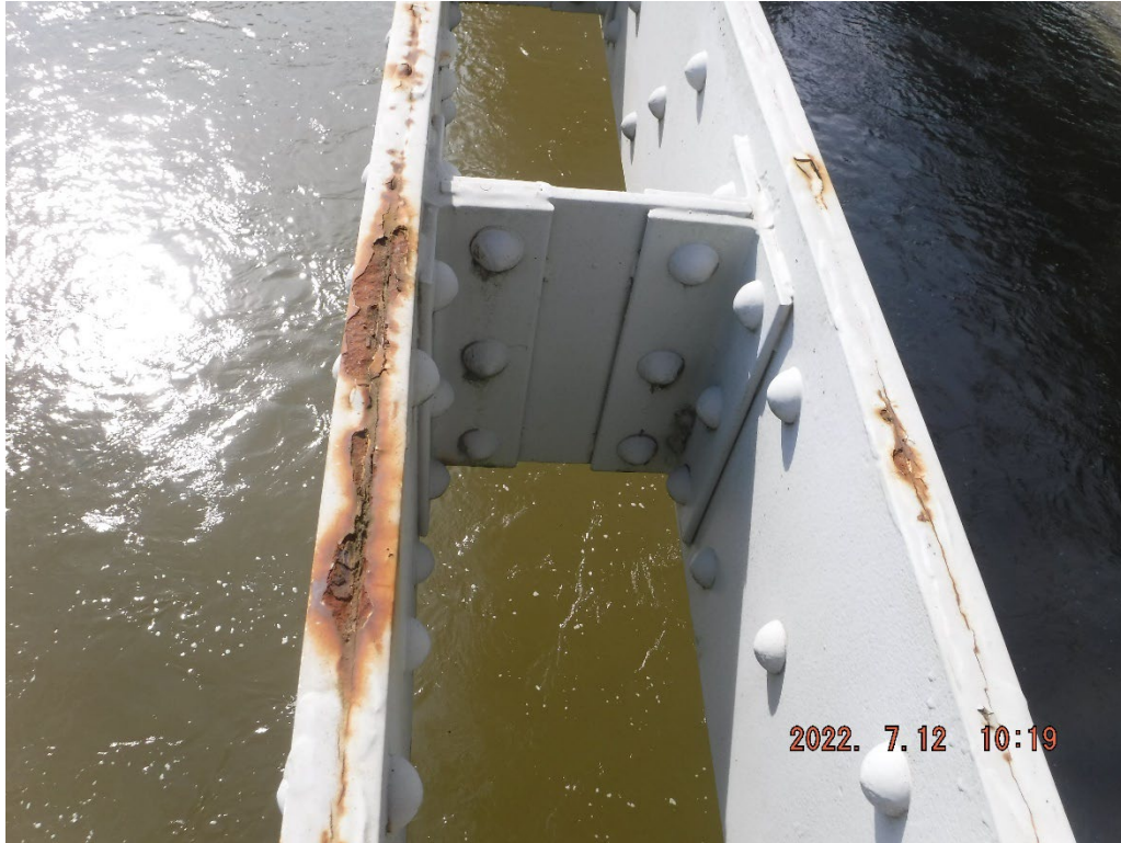
Photo 19: Active pitting on plate edges, L3L4, Span 1, North Truss
