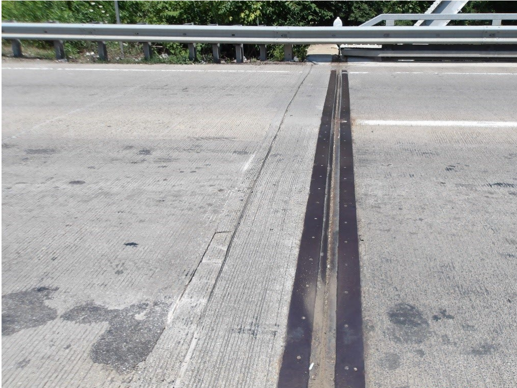
Photo 80: Asphalt patches and longitudinal cracks in Rear Approach Slab near abutment joint
