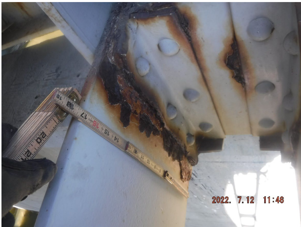
Photo 22: Active laminating corrosion with section loss up to 1/8" deep x full plate width on L0L1 at L0, Span 2, North Truss
