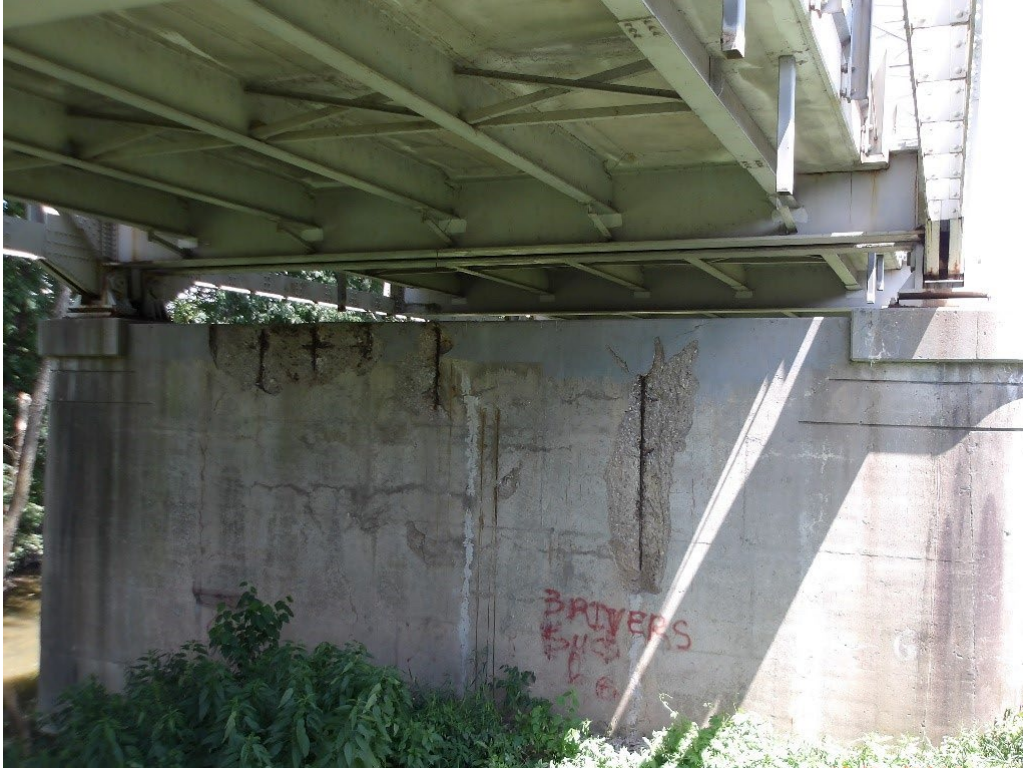
Photo 71: Widespread spalls with exposed rebar on the west face of Pier 4
