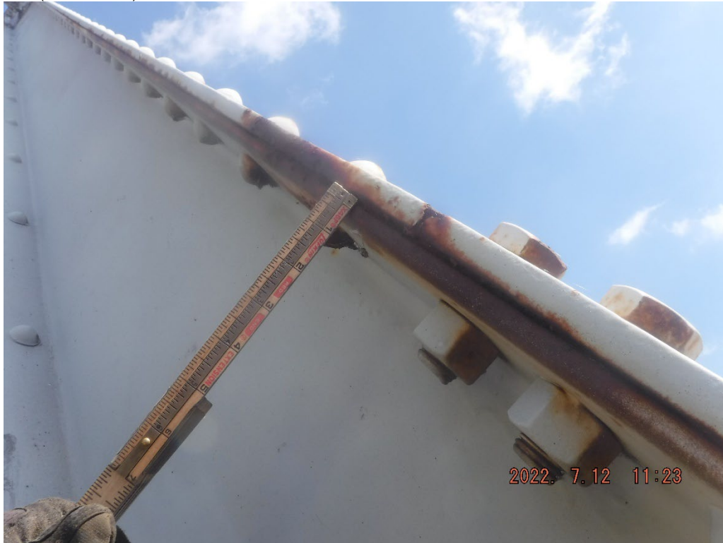
Photo 28: Active pack rust up to 1/8" thick in U7L8, Span 1, North Truss
