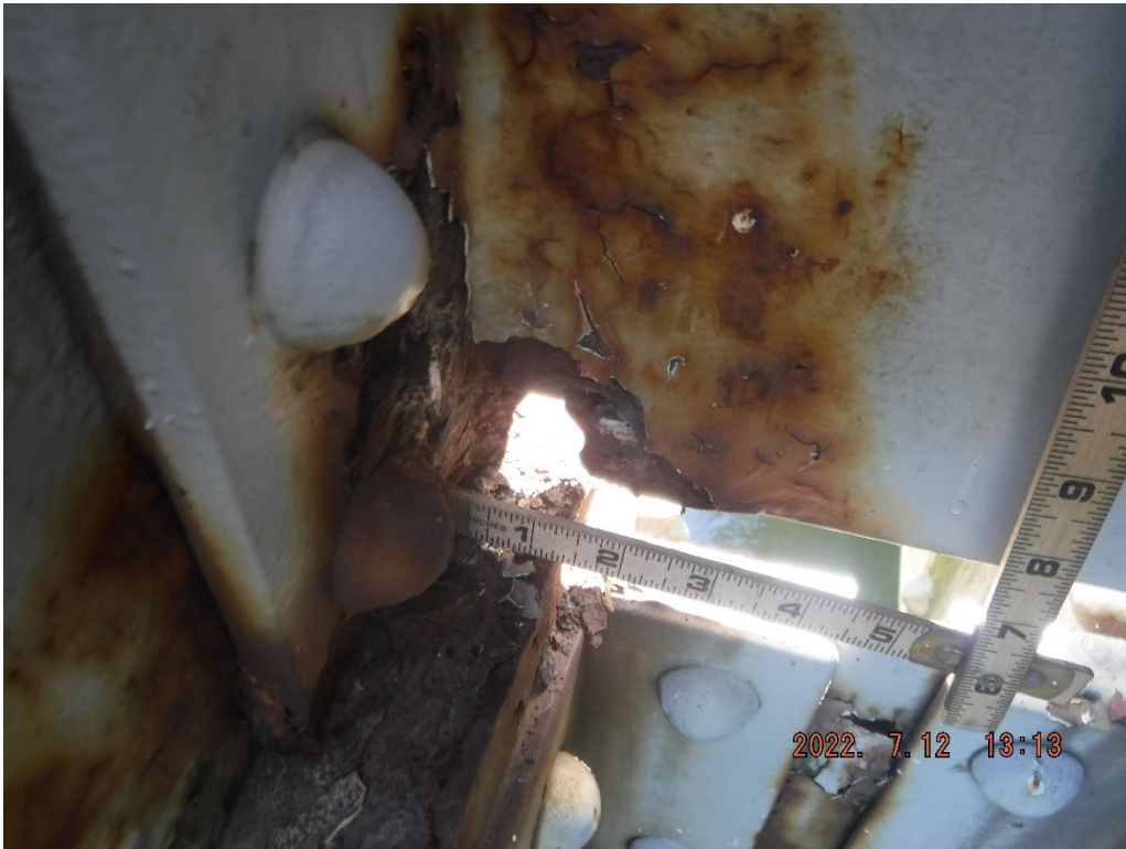
Photo 34: 1" Diameter corrosion hole at L6U6, Span 2, North Truss
