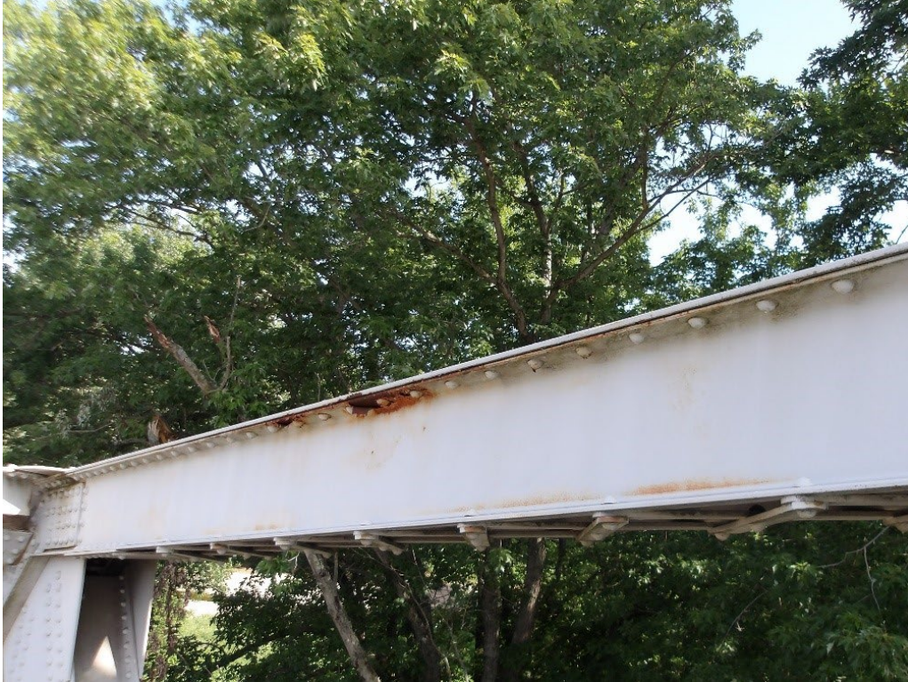
Photo 26: Active corrosion on U1U2, Span 4, North Truss
