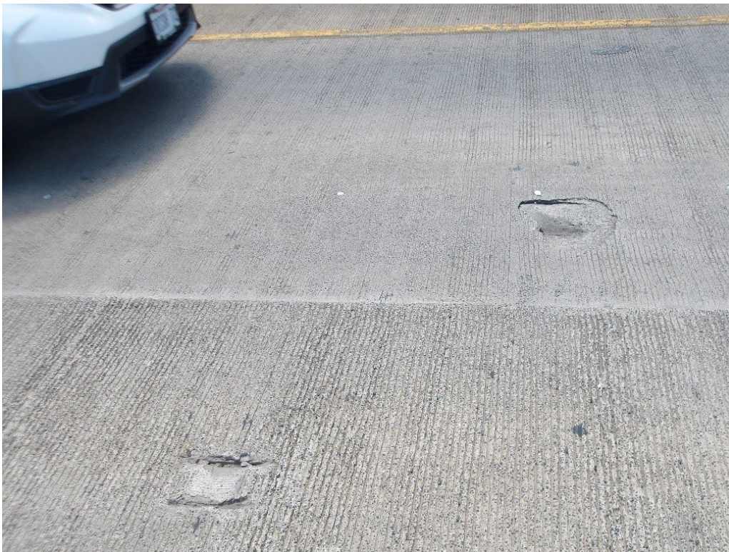
Photo 8: Missing RPM and 4 S.F. spall in south lane in Span 3
