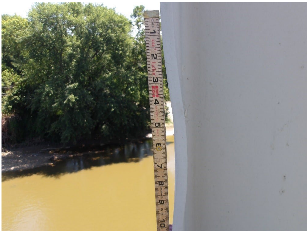
Photo 36: Bowing of outboard flange of L7U7, Span 4, North Truss
