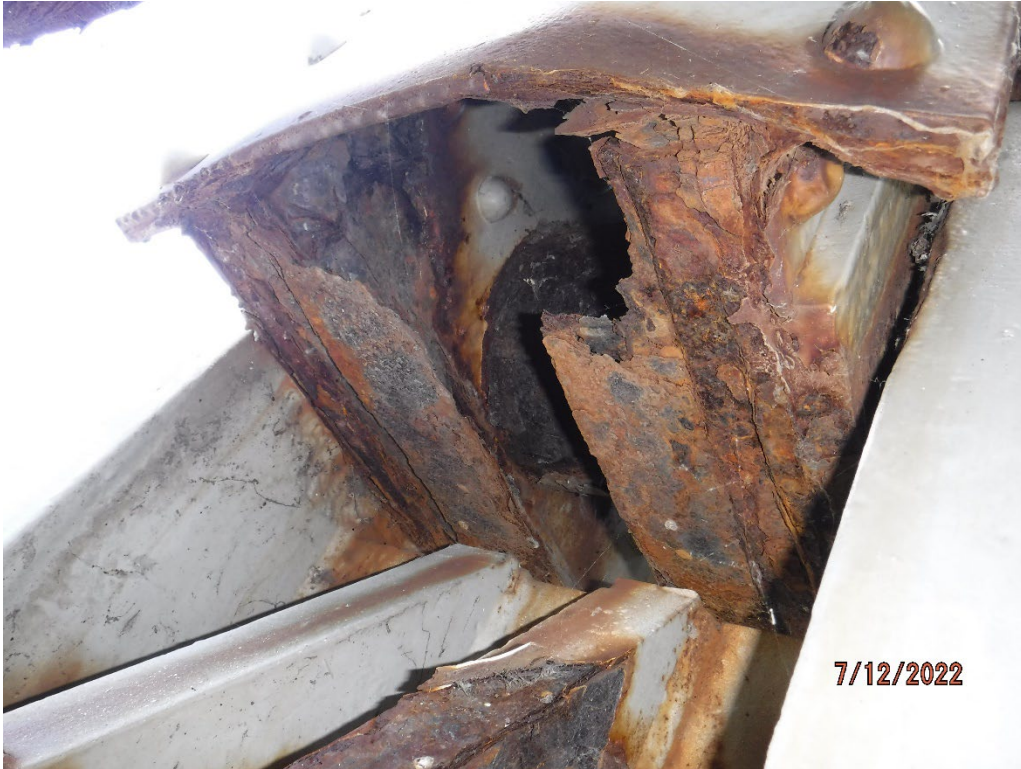
Photo 52: Corrosion holes in L0 gusset plate stiffening angles and bowed side cover plate behind Pier 2 bearing, Span 2, North Truss
