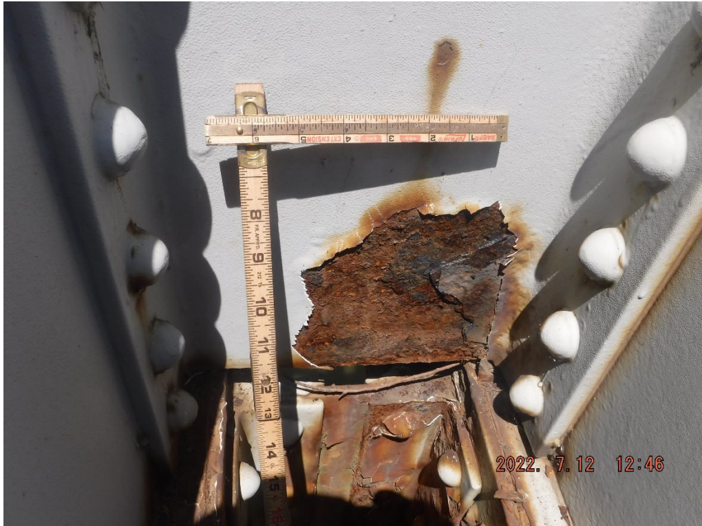
Photo 32: Active pitting with section loss up to 1/16" deep at L3U3 on Span 2, North Truss
