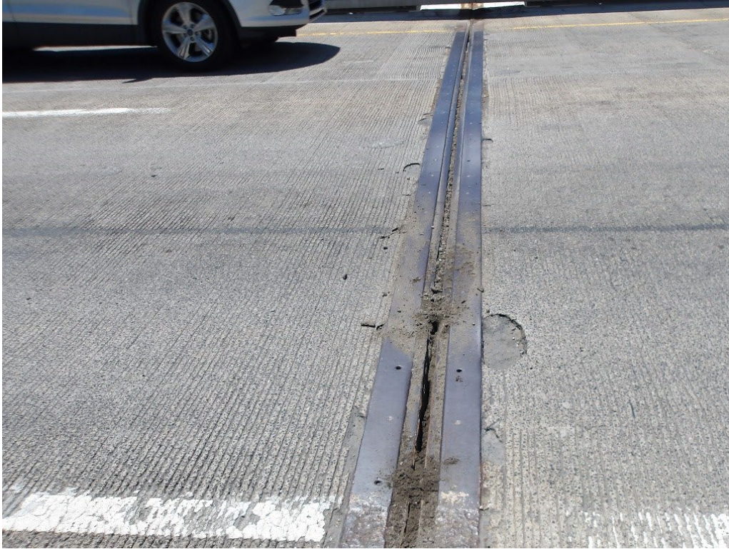
Photo 7: Isolated spalls adjacent to Pier 2 joint
