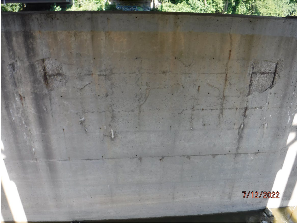
Photo 69: Delaminations and spalls with exposed rebar on east face of Pier 2
