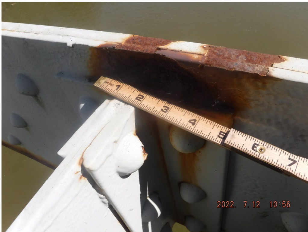
Photo 20: Active pitting up to 3/16" deep at L5L6, Span 1, North Truss
