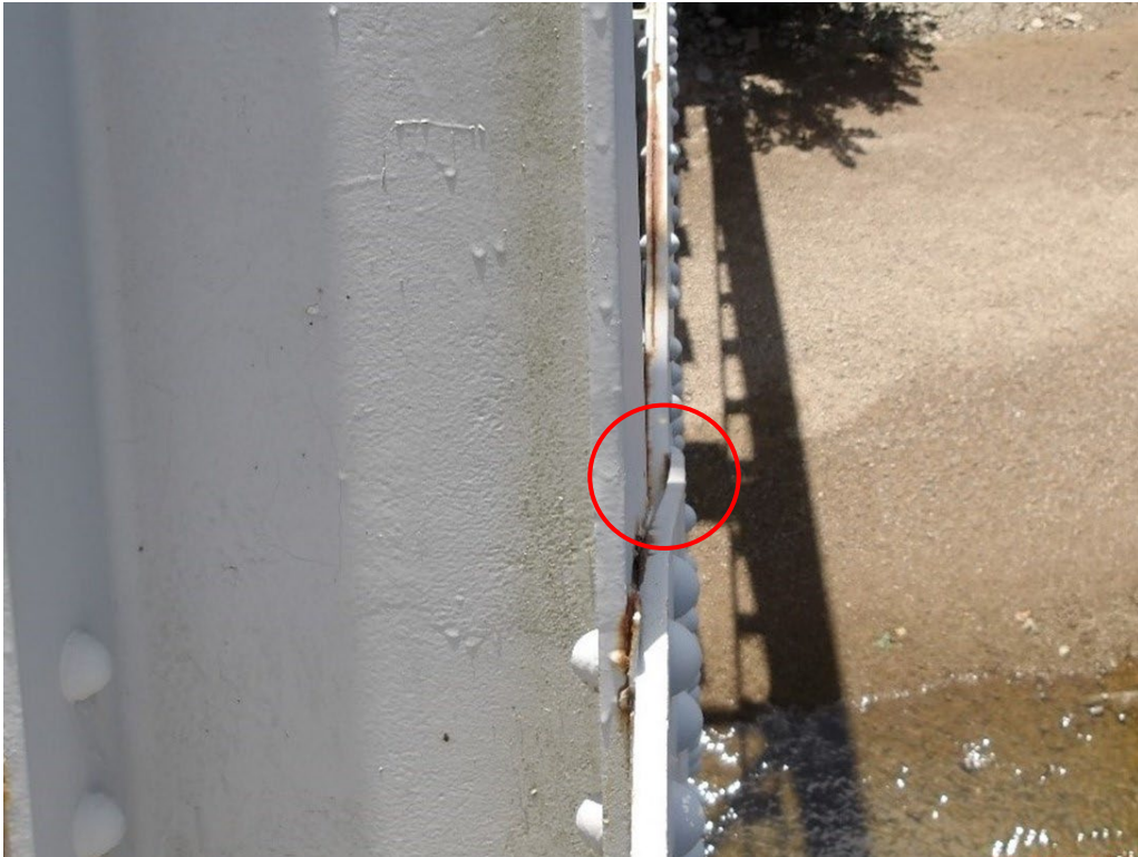
Photo 57: Positive bowing on outboard gusset plate L7, Span 2, South Truss
