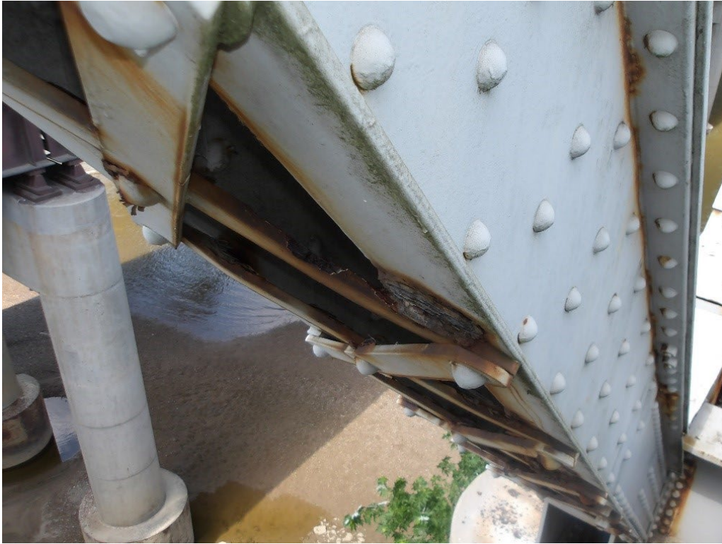
Photo 30: Pack rust up to 3/16" thick under lacing bars of LOU1, Span 3, South Truss
