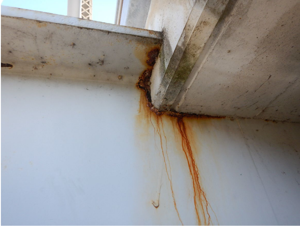
Photo 45: Typical corrosion on top flange and web at the deck penetration at FB 9, Span 2, South end
