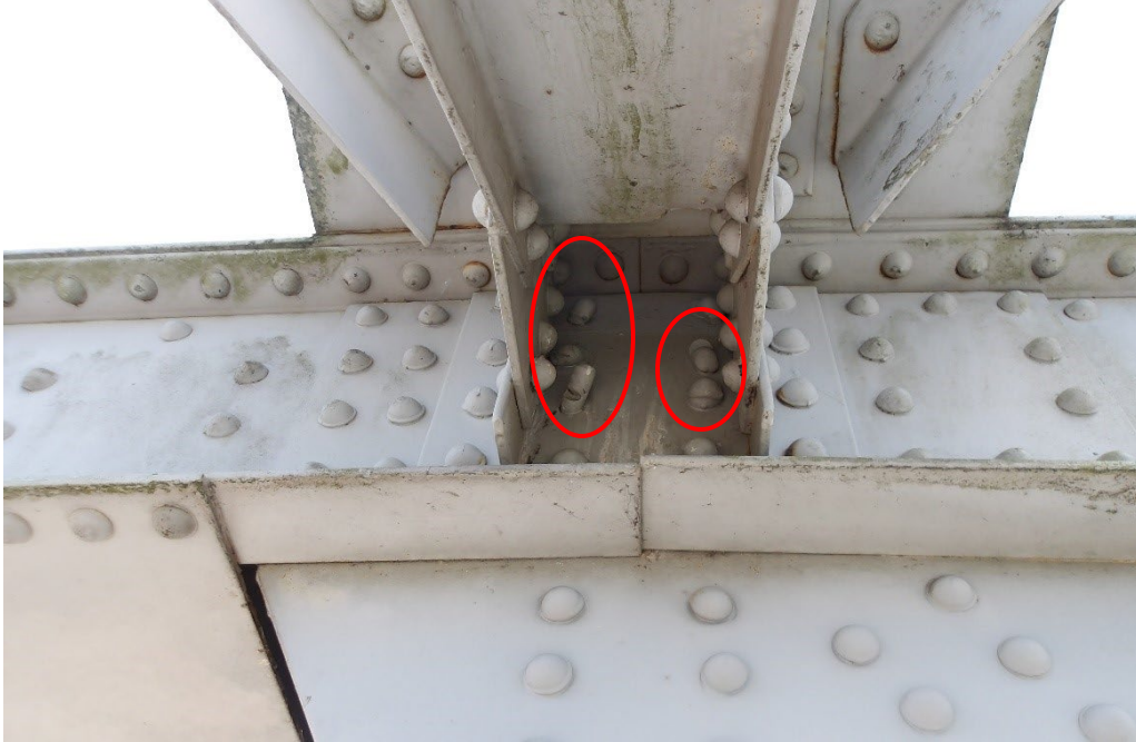
Photo 50: Improperly installed rivets at U6, Span 2, South Truss
