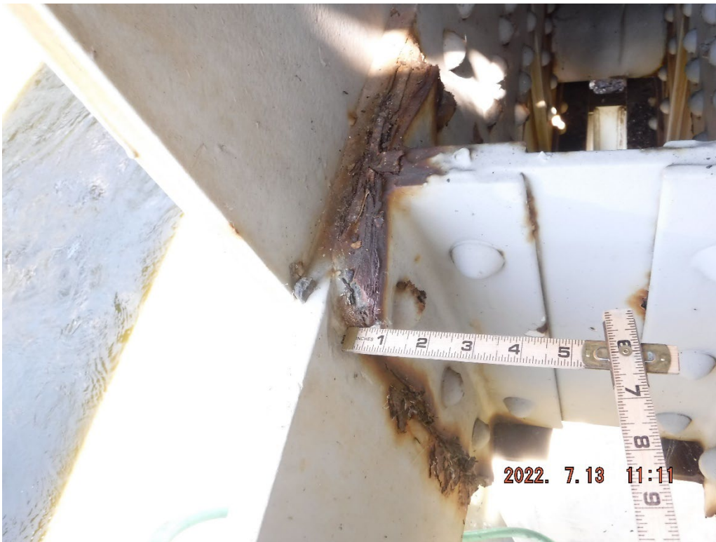
Photo 18: Pack rust up to 3/4" thick at LOL1, Span 2, South Truss
