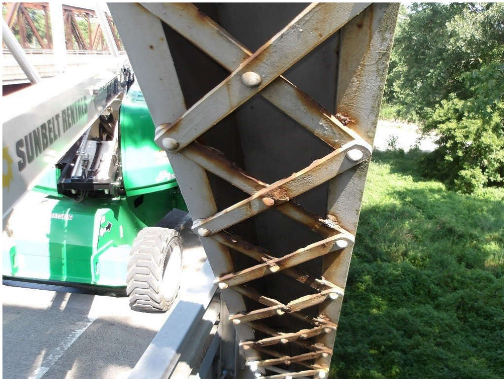
Photo 29: Active corrosion with section loss up to 1/8" deep on lacing of LOU1, Span 4, North Truss
