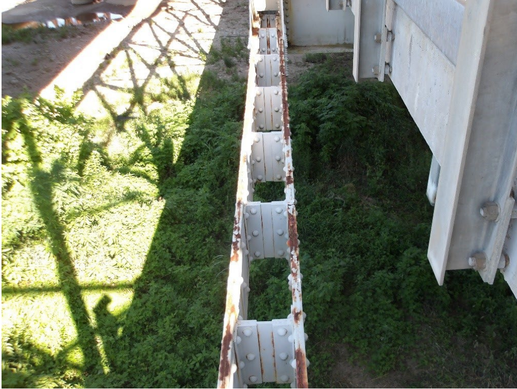
Photo 15: Typical pack rust between lower chord plates (L6L7, Span 3, South Truss shown)
