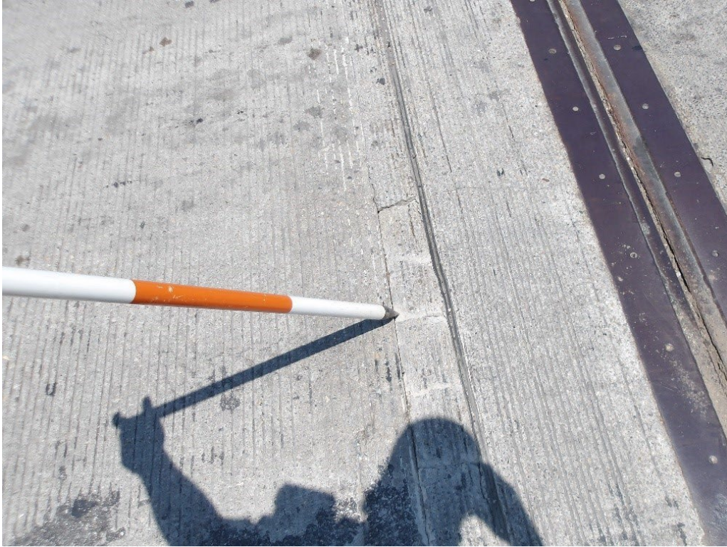
Photo 81: 3 S.F. of cracking with broken up concrete in Rear Approach Slab adjacent to abutment joint
