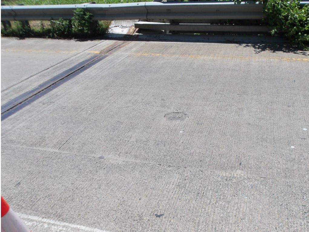
Photo 9: 1 S.F spall near centerline of Span 4
