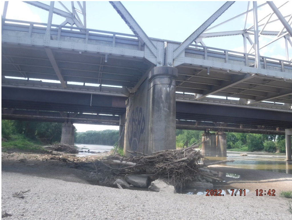
Photo 84: Scour and debris around Pier 3
