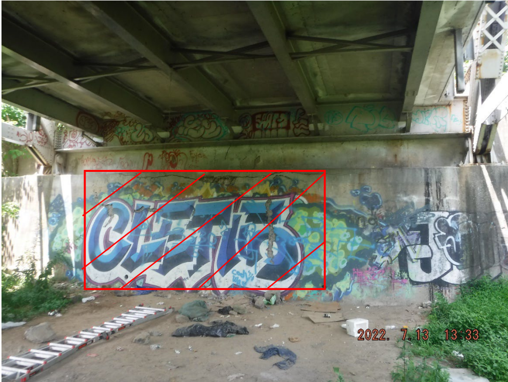
Photo 72: Extents of delaminations on Rear Abutment
