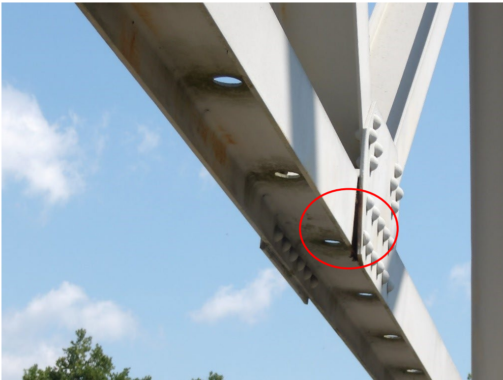
Photo 67: Warped sway brace gusset plate at PP4 in Span 3
