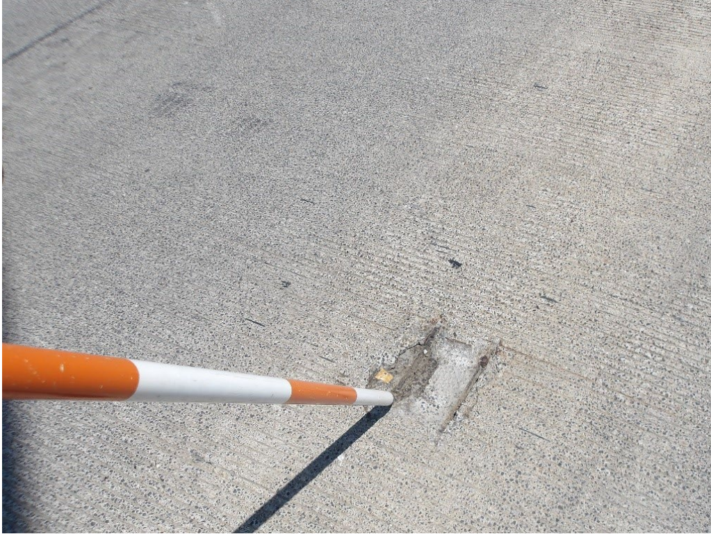
Photo 5: Missing RPM in Span 1
