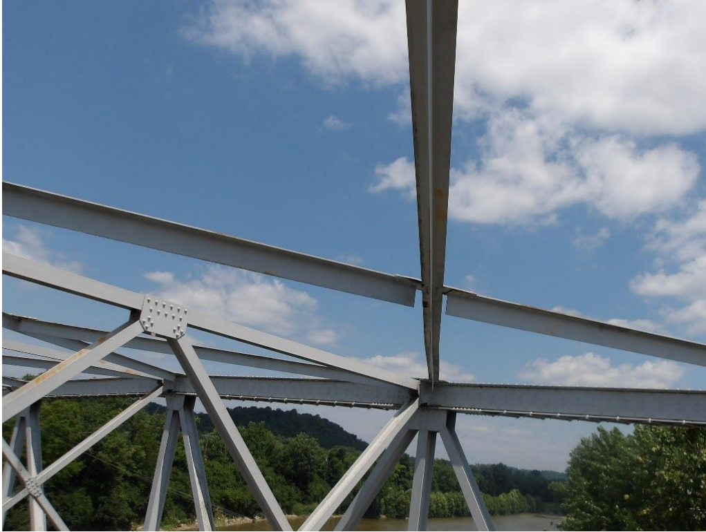
Photo 65: Bent lateral bracing at U5U6 on Span 2
