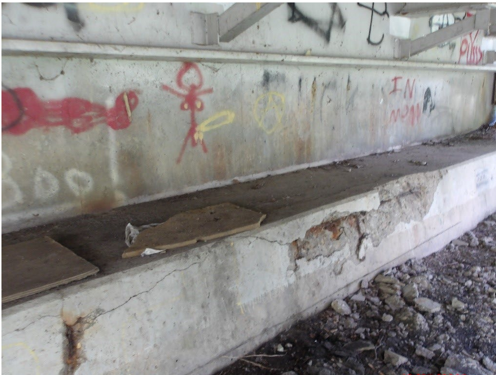
Photo 75: Spalls with exposed rebar at Forward Abutment
