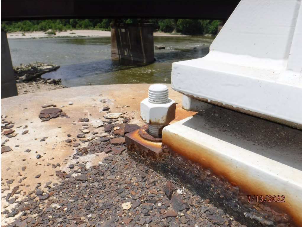
Photo 61: Loose southeast anchor nut at South bearing, Span 2, Pier 3
