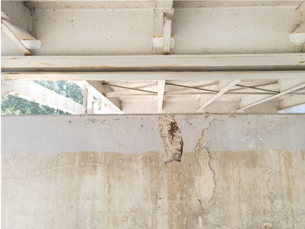
Photo 77: Spall with exposed rebar on west face of Pier 3 cap
