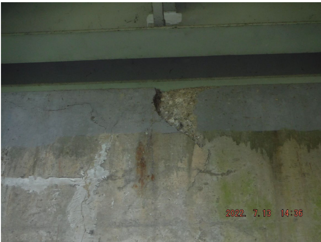
Photo 78: Spall on east face of Pier 4 cap
