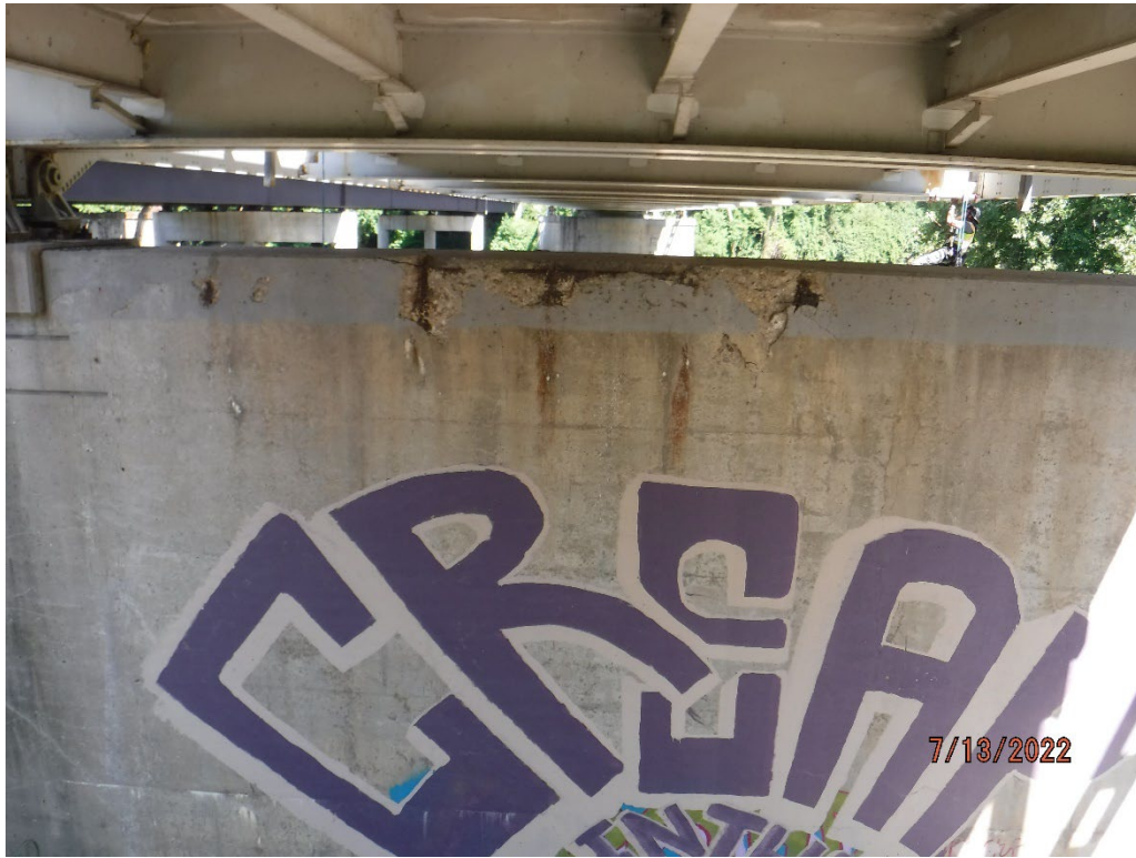
Photo 76: Spall with exposed rebar on east face of Pier 3 cap
