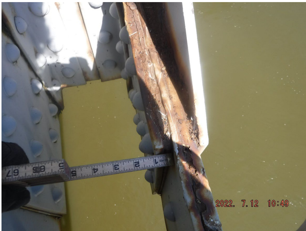
Photo 49: Active pack rust up to 3/8" thick at L5 splice plate, Span 1, North Truss
