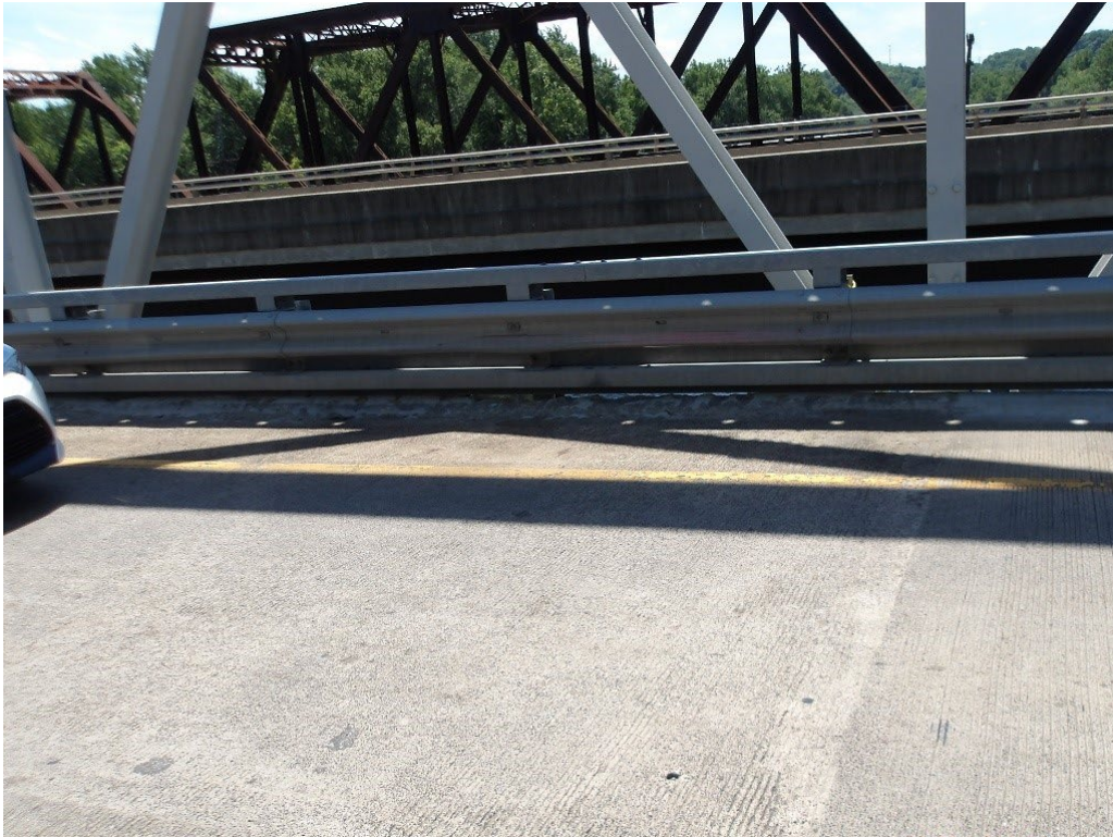
Photo 11: Curb spall at south railing in Span 2
