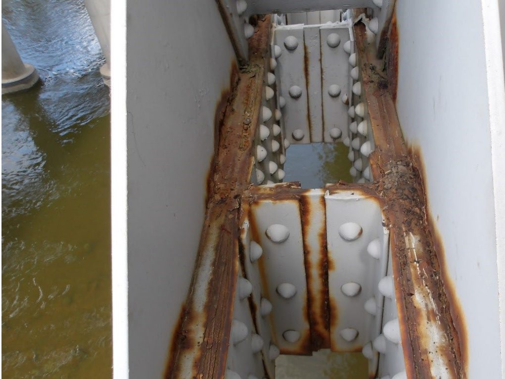
Photo 17: Active pack rust at L7, Span 2, South Truss
