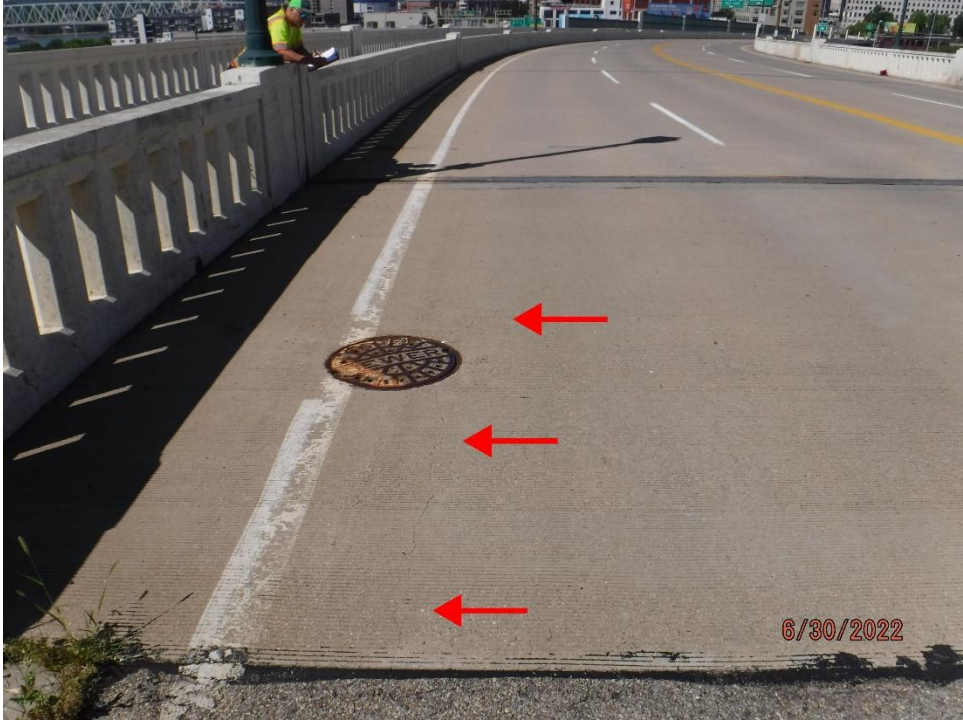
Photo 97: East Approach Slab with cracks propagating from drainage structure
