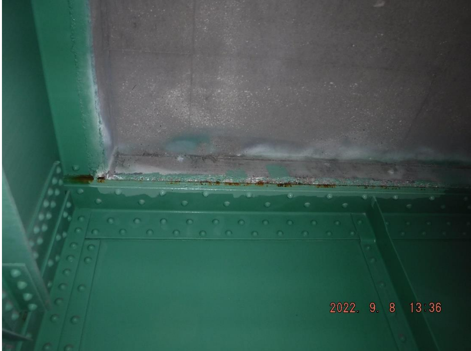
Photo 48: Example of laminar corrosion between the floor beam and concrete haunch (Span 1 shown)
