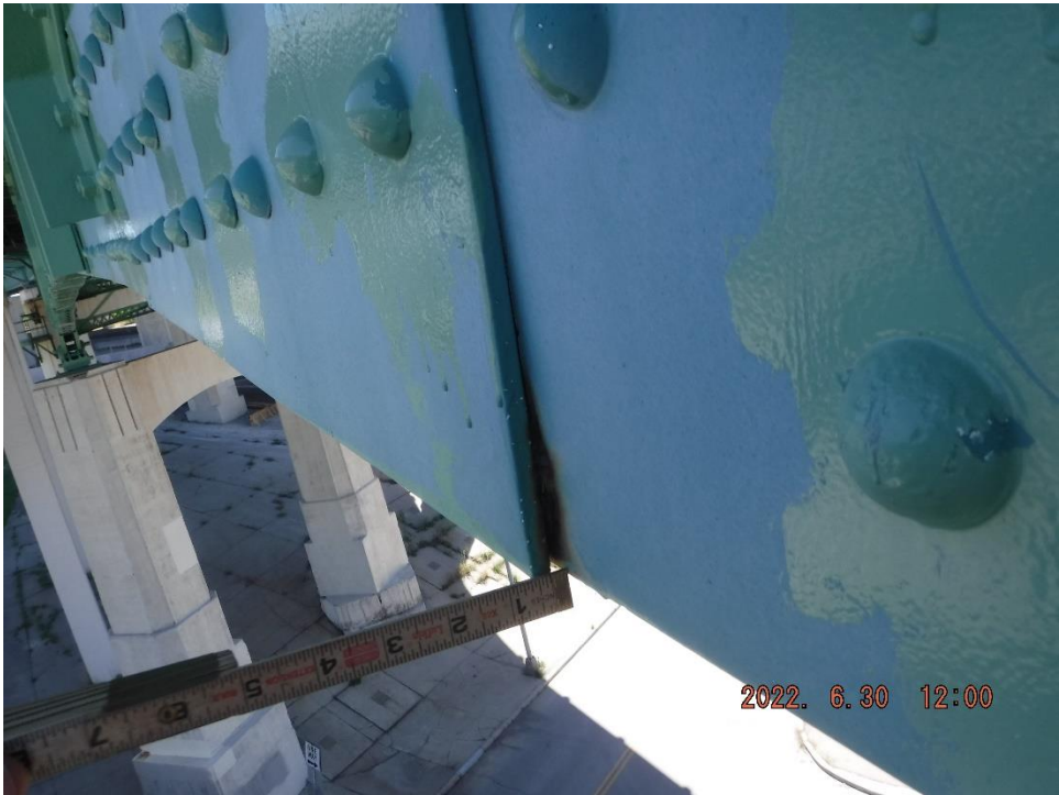
Photo 27: Example of splice plate separation due to pack rust (North face of North Truss, Span 10, at L16 shown)
