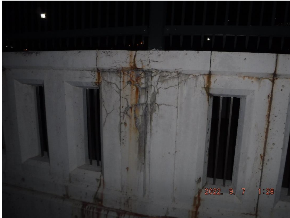
Photo 10: Cracking and rust staining on exterior face of bridge railing (South Railing, Span 9 shown)
