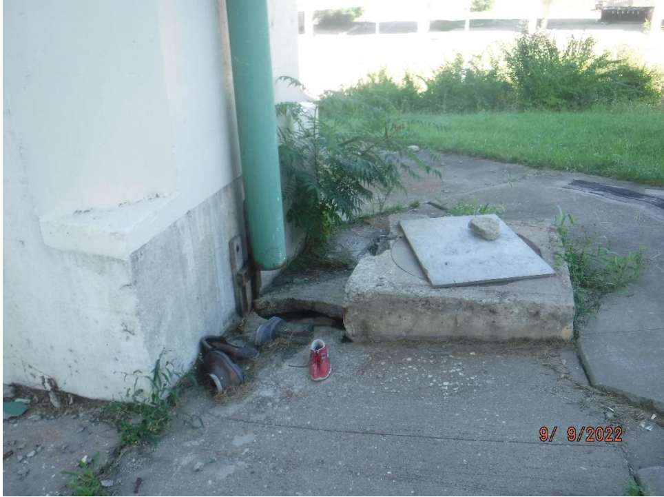
Photo 14: Example of broken ground termination and undermining of the slope protection (Column 1 at Pier 12 shown)
