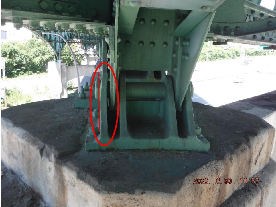
Photo 70: Bent pin support plate at Pier 10, Center Truss, Span 10 Bearing
