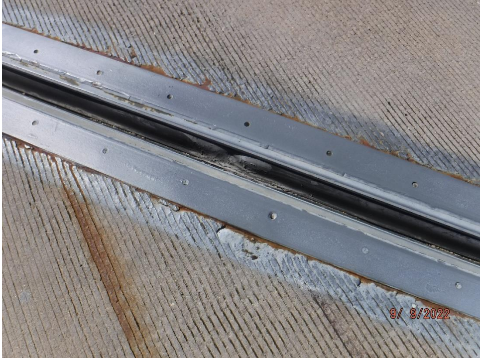
Photo 8: Tear in expansion joint seal material (Pier 7 shown)
