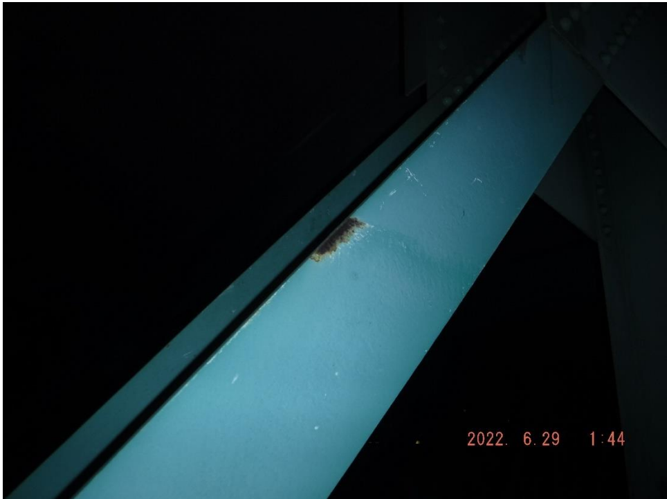
Photo 44: Active surface corrosion on the flange of U20-L21 in Span 8 of the North Truss
