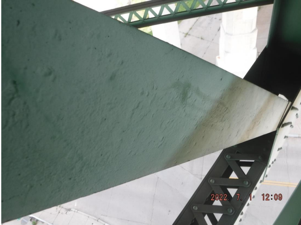
Photo 43: Painted-over pitting on the member flange (Center Truss, Span 10, L15-U16 shown)
