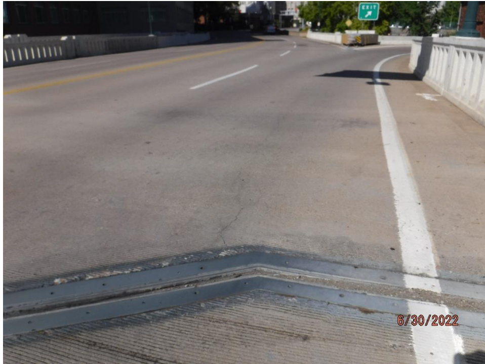
Photo 5: Wearing surface with typical cracks
