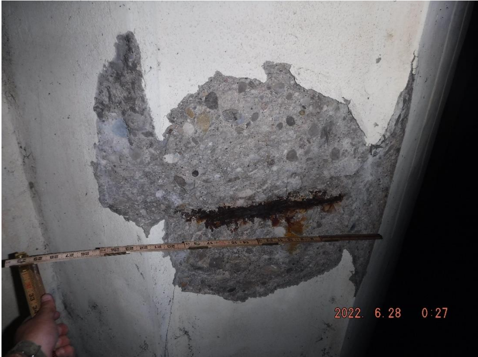
Photo 85: Spall with exposed reinforcement on the Center Column of Pier 13
