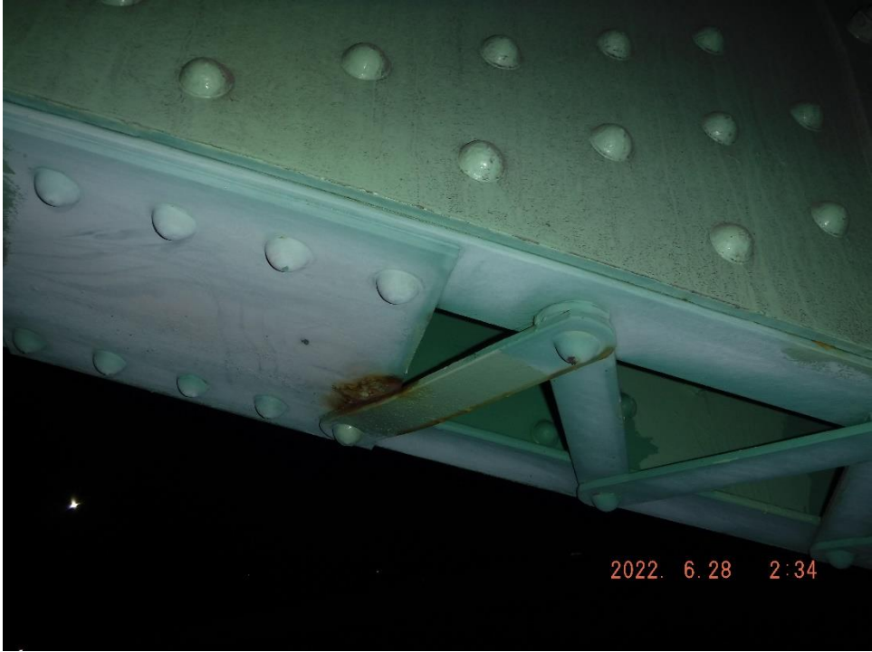
Photo 28: Example of surface corrosion on lacing bar and tie plate (North Truss, Span 9 at L43 shown)
