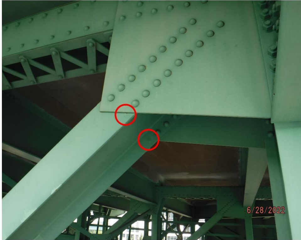
Photo 45: Mis-drilled holes in the member flange filled with plug welds at U3 on U3-L4 in Span 5 of the North Truss
