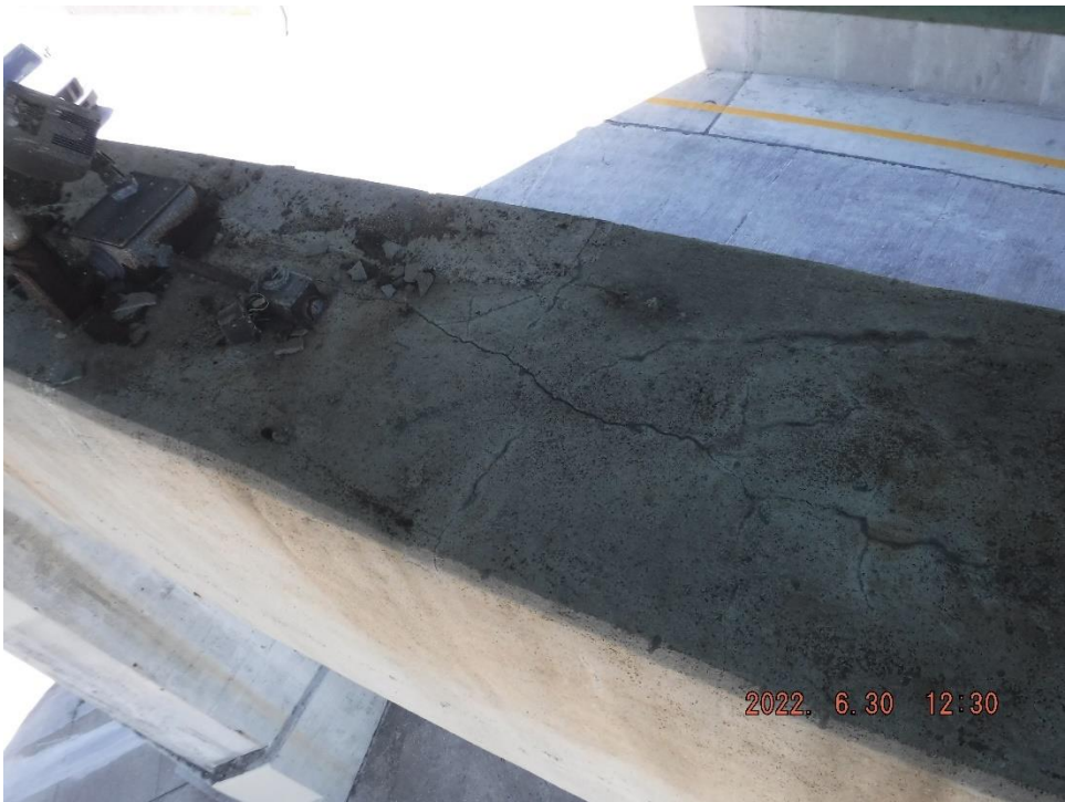
Photo 93: Map cracking on the top face of the Pier 10 Cap between the Center and South Columns
