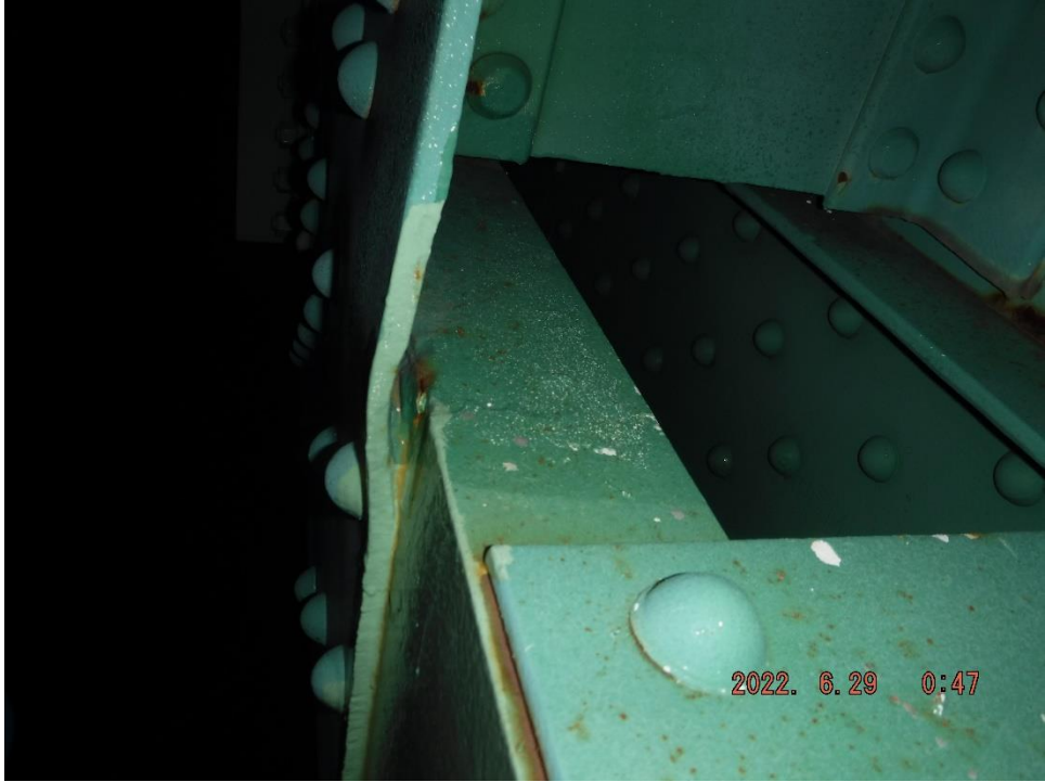
Photo 63: Free edge localized deformation with pack rust at unrepaired gusset edge (Span 8, North Truss, L25, North Gusset shown)
