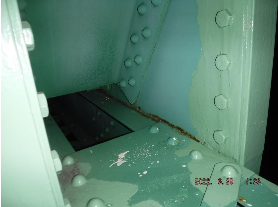
Photo 56: Laminar corrosion along member flange on inside face of gusset plate (Span 8, North Truss, L19, South Gusset shown)
