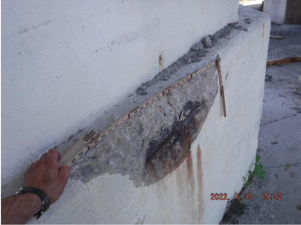
Photo 84: Spall with exposed reinforcement on the Center Column of Pier 13
