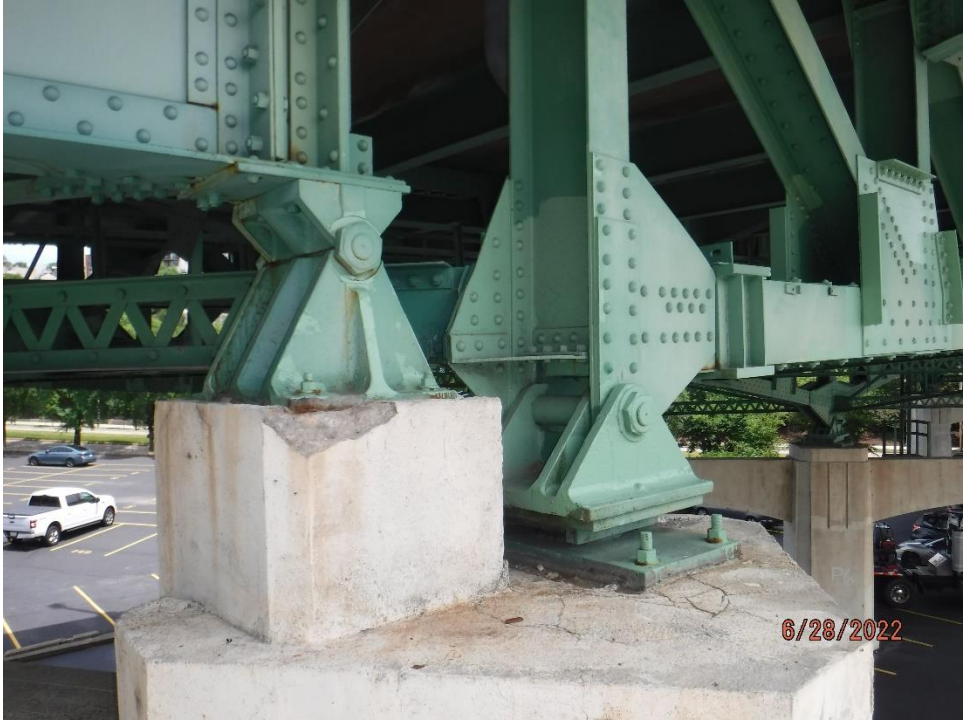
Photo 90: 1' x 6" spall beginning to undermine the Span 4 Bearing of the South Truss at Pier 5
