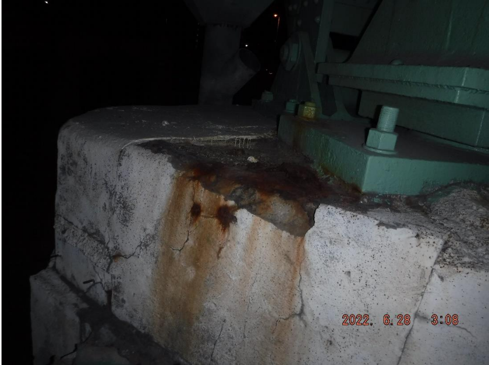
Photo 92: Spall beginning to undermine the Span 9 Bearing at the South Truss at Pier 10
