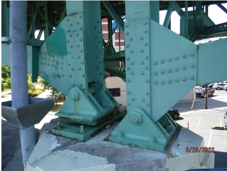
Photo 68: Painted-over pitting and surface corrosion on bearings (North Truss at Pier 7 shown)
