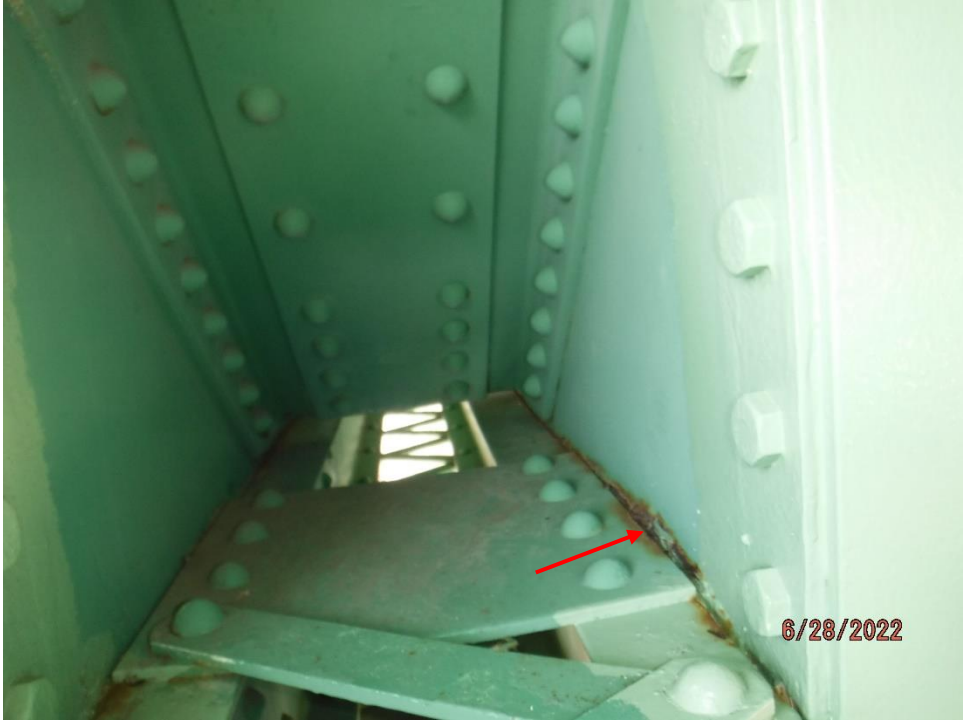
Photo 52: Reactivating pack rust between gusset and lower chord (Span 5, North Truss, L1, South Gusset shown)
