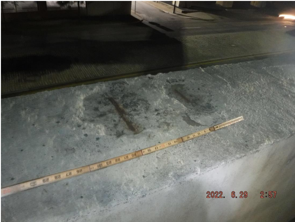
Photo 91: 2' x 1' spall with exposed reinforcement on the top face of Pier 8 Cap between the Center and South Columns
