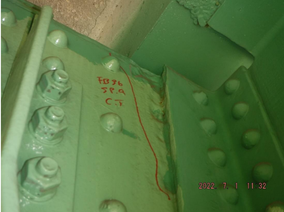
Photo 54: Painted-over pitting on gusset plate at floor beam connection (Span 9, Center Truss, U36, South Gusset shown)
