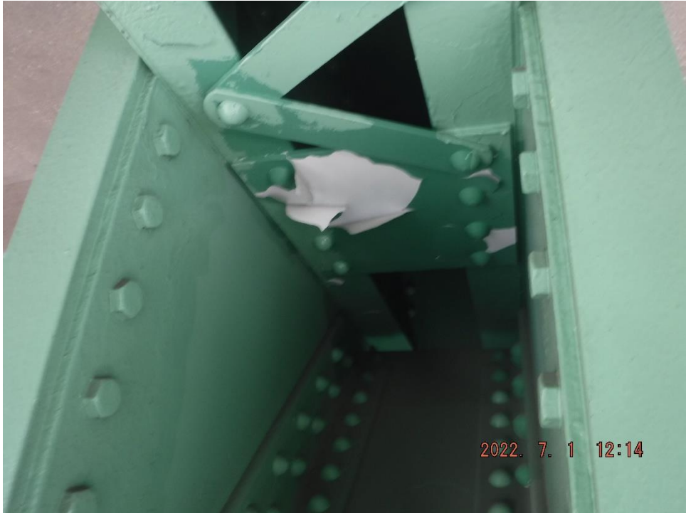
Photo 78: Example of peeling paint (upper chord tie plate shown)
