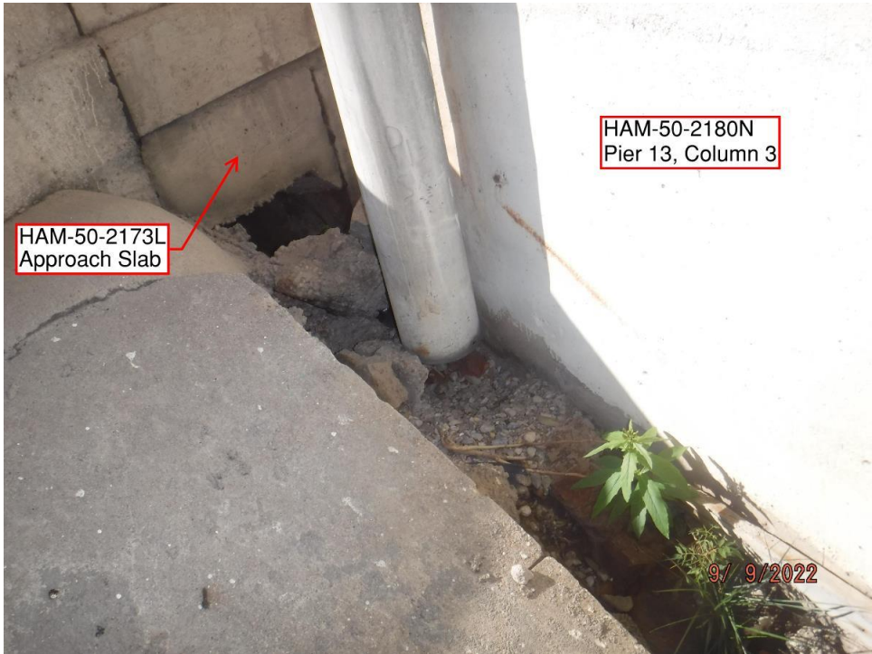
Photo 15: Broken ground termination and undermining of approach slab of adjacent structure (HAM-50-2173L) at Column 3 of Pier 13
