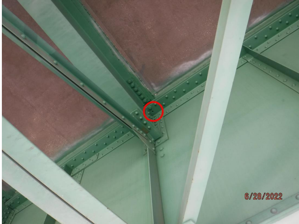
Photo 50: Mis-drilled hole in built-up girder beam top flange at floor beam connection (Span 4, North Girder, Floor Beam 5 shown)
