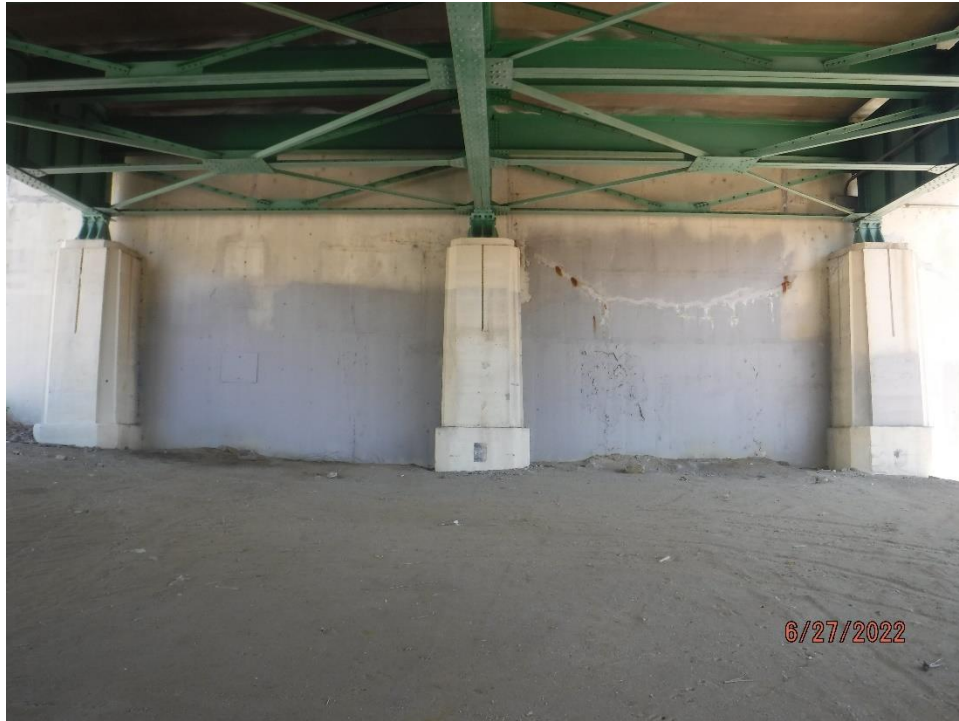
Photo 89: Sealed horizontal crack and map cracking on the Forward Abutment
