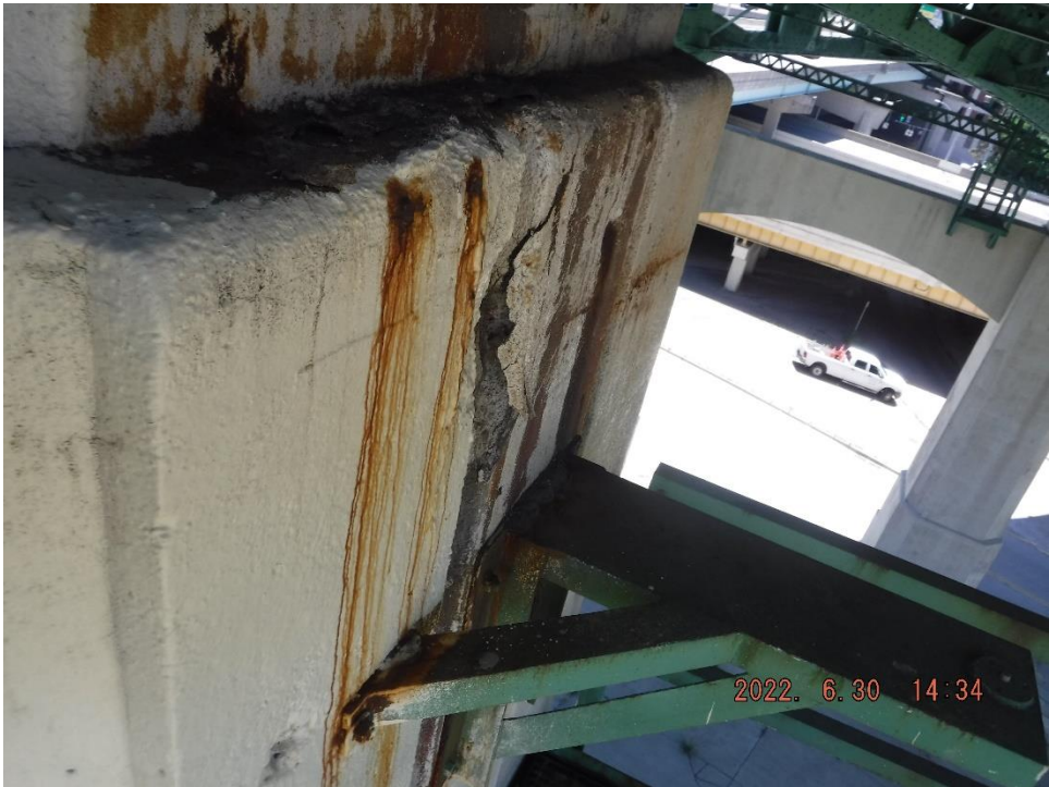
Photo 83: Spall with rust staining on the North Column of Pier 12
