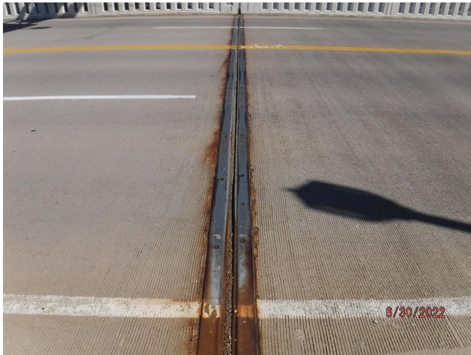
Photo 7: Typical expansion joint surface corrosion and debris fill (Pier 13 shown)
