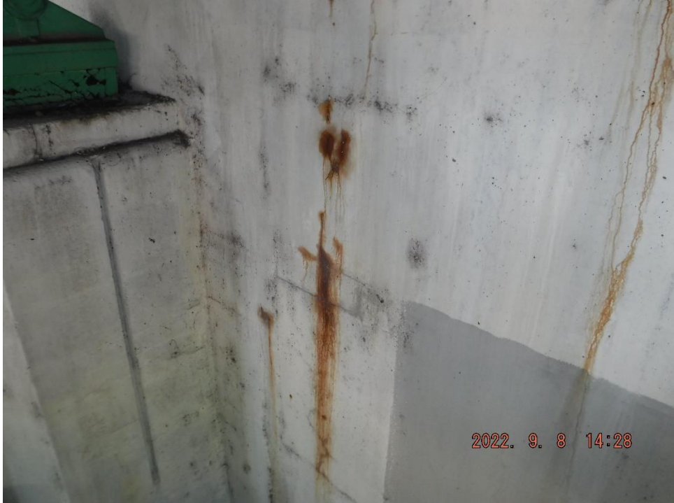
Photo 87: Hairline map cracking with rust staining on the Rear Abutment
