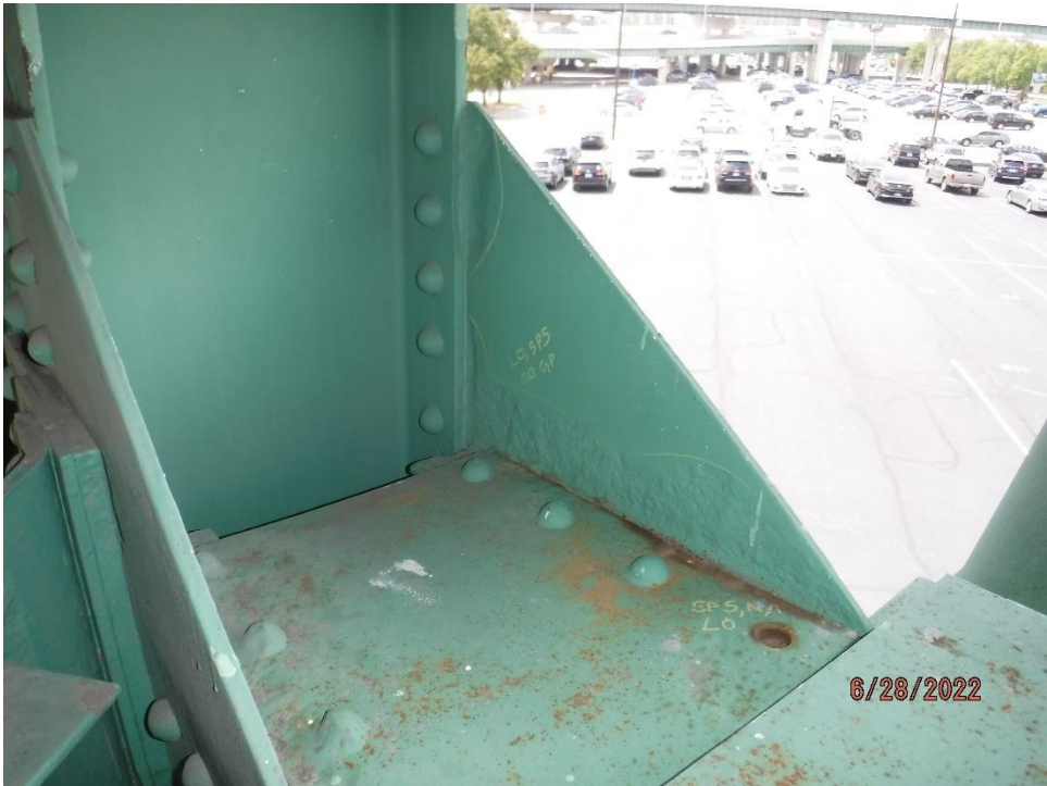
Photo 55: Painted-over pitting on inside face of gusset plate (Span 5, North Truss, L0, North Gusset shown)
