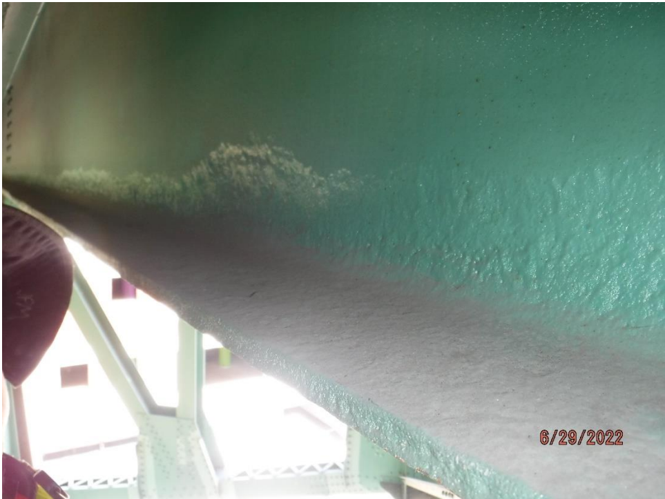
Photo 47: Painted-over section loss in floor beam web and bottom flange (Center Truss, Span 6 South bay, at U20 shown)
