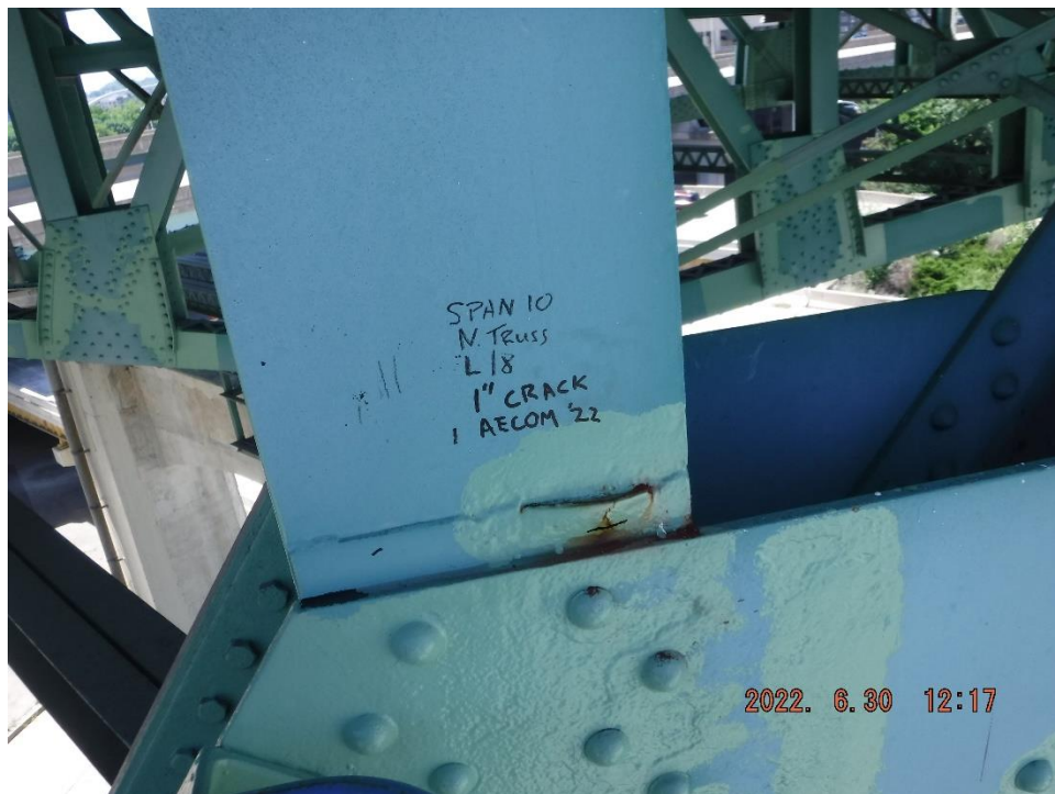
Photo 39: Active pack rust behind cracked tack weld and fill plate (North Truss, Span 10, L18-U18 shown)
