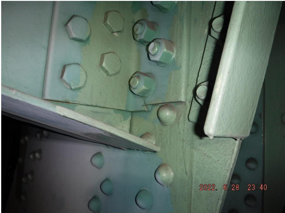
Photo 49: Field cut cantilever bracket connection angle (Span 8, South Truss at U27 shown)
