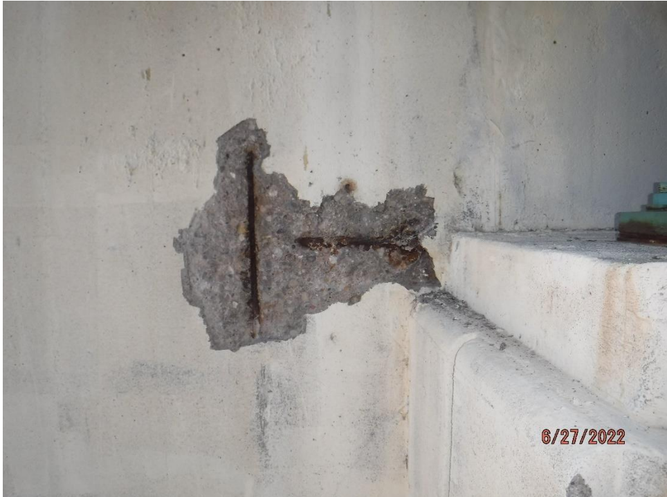
Photo 88: 2 SF spall with exposed reinforcement adjacent to the North Girder on the Forward Abutment
