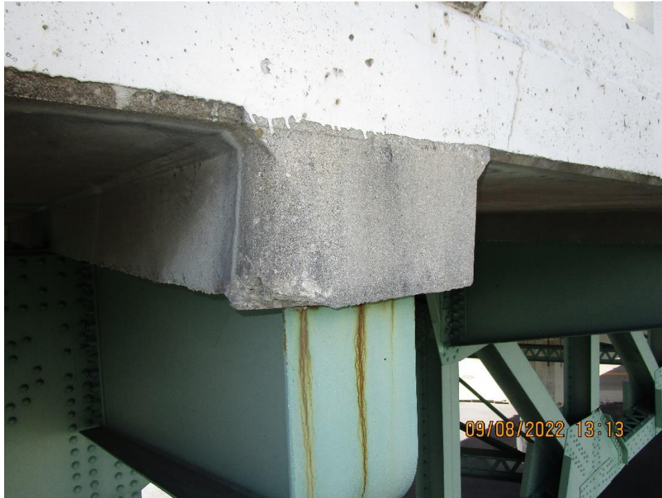
Photo 3: Example of haunch before the delaminated concrete was removed (Bracket 9 at Pier 6 shown)
