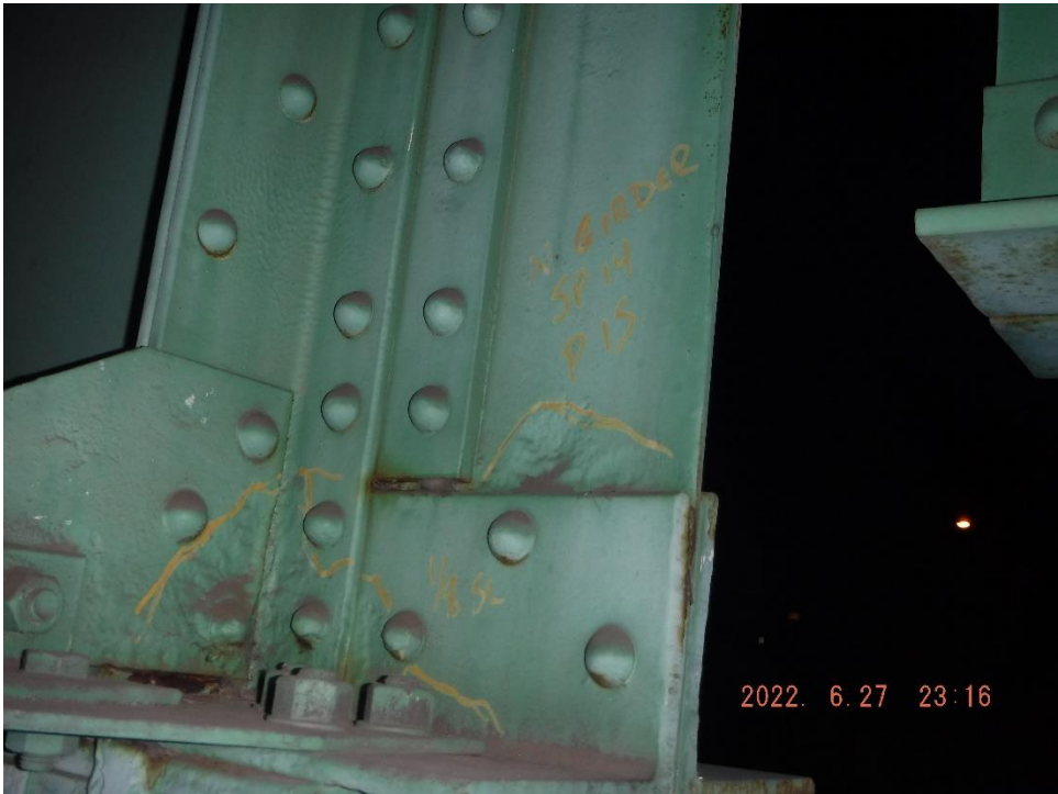
Photo 20: Example of painted-over pitting (North Girder, Span 14 at Pier 15 shown)
