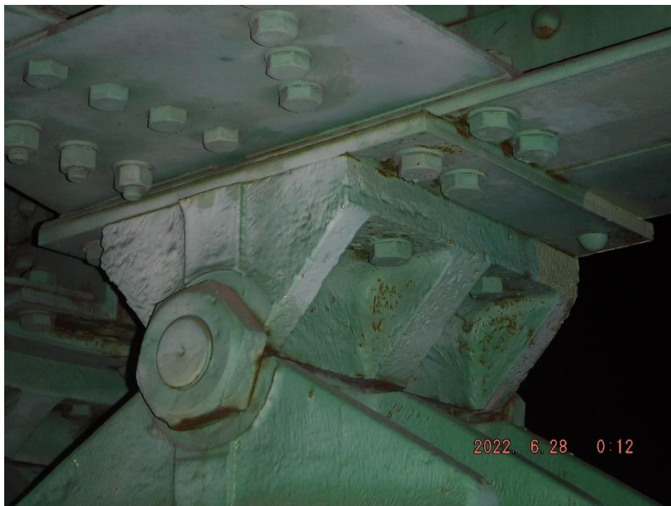
Photo 69: Painted-over pitting on bearing (North Girder, Span 13, at Pier 13 shown)
