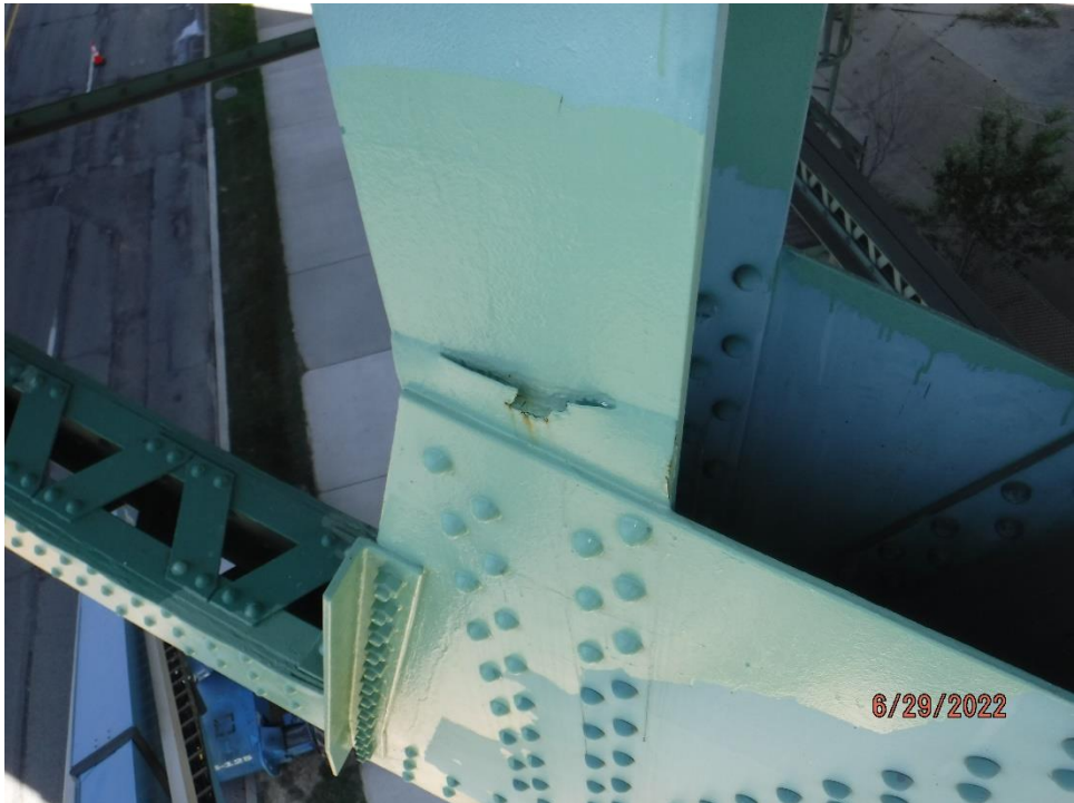
Photo 37: Fill plate cracked and deformed due painted-over pack rust between fill plate and member (South Truss, Span 7, L13-U13 shown)
