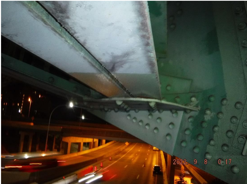
Photo 81: Bent bracing member gusset at L32 on Span 9 of the South Truss
