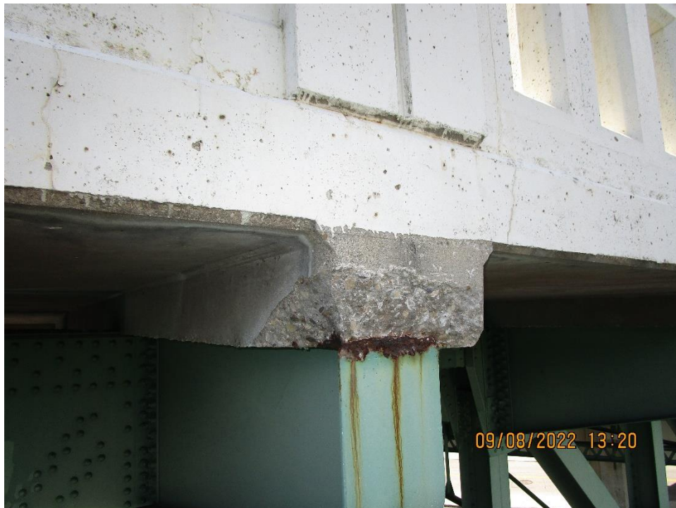
Photo 4: Example of haunch after the delaminated concrete was removed (Bracket 9 at Pier 6 shown)
