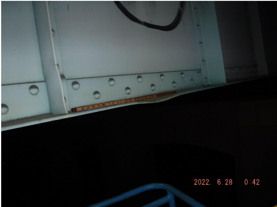
Photo 24: 1/2" out of plane bending of bottom flange on the South Girder in Span 12 near midspan
