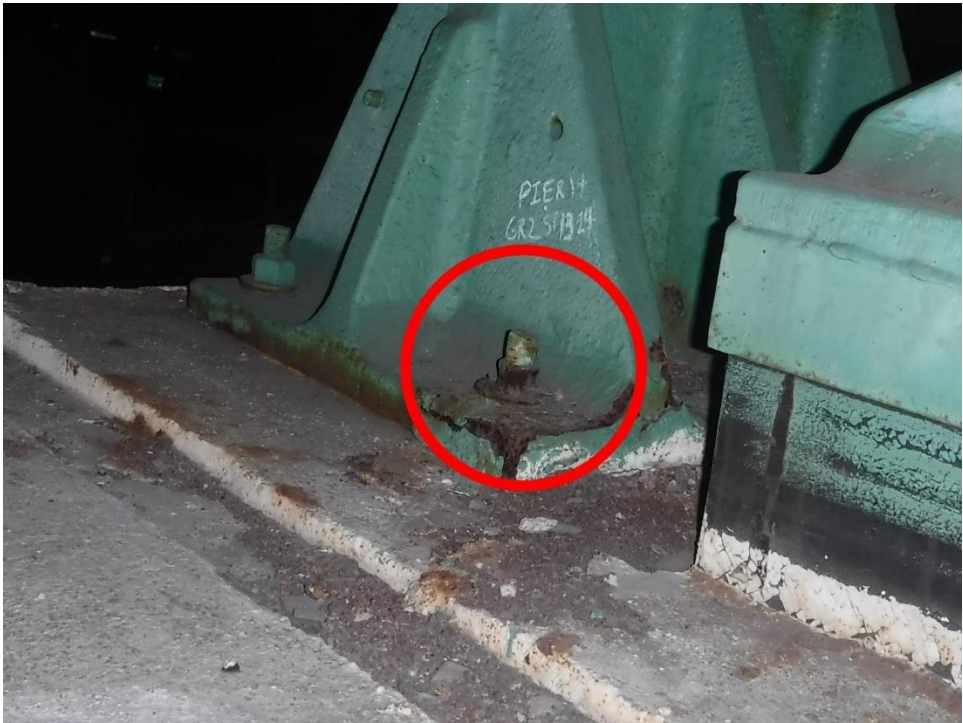
Photo 73: Section loss on anchor nut at Pier 14, Center Girder, Span 13
