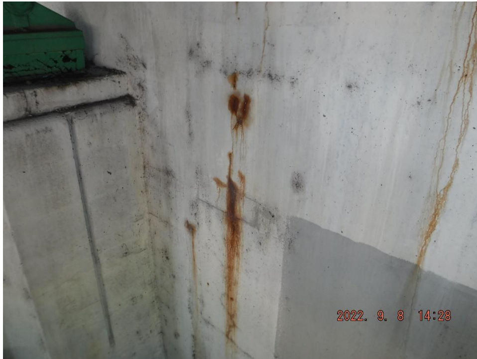
Photo 96: Cracks with efflorescence and rust staining on the rear abutment backwall
