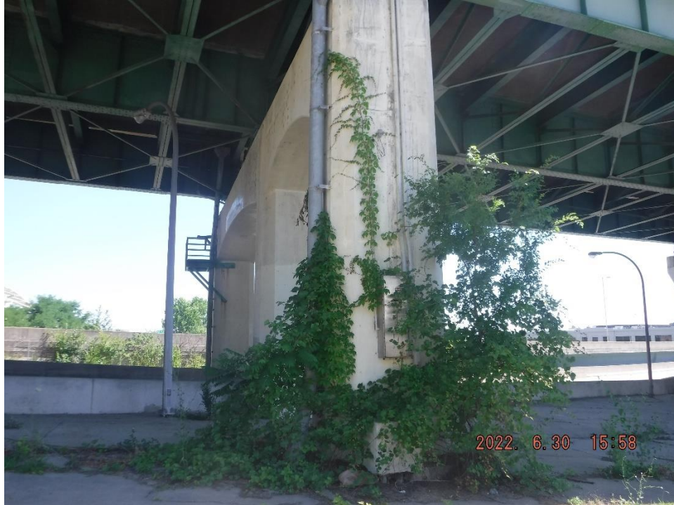
Photo 86: Vegetation growing on the North Column of Pier 14
