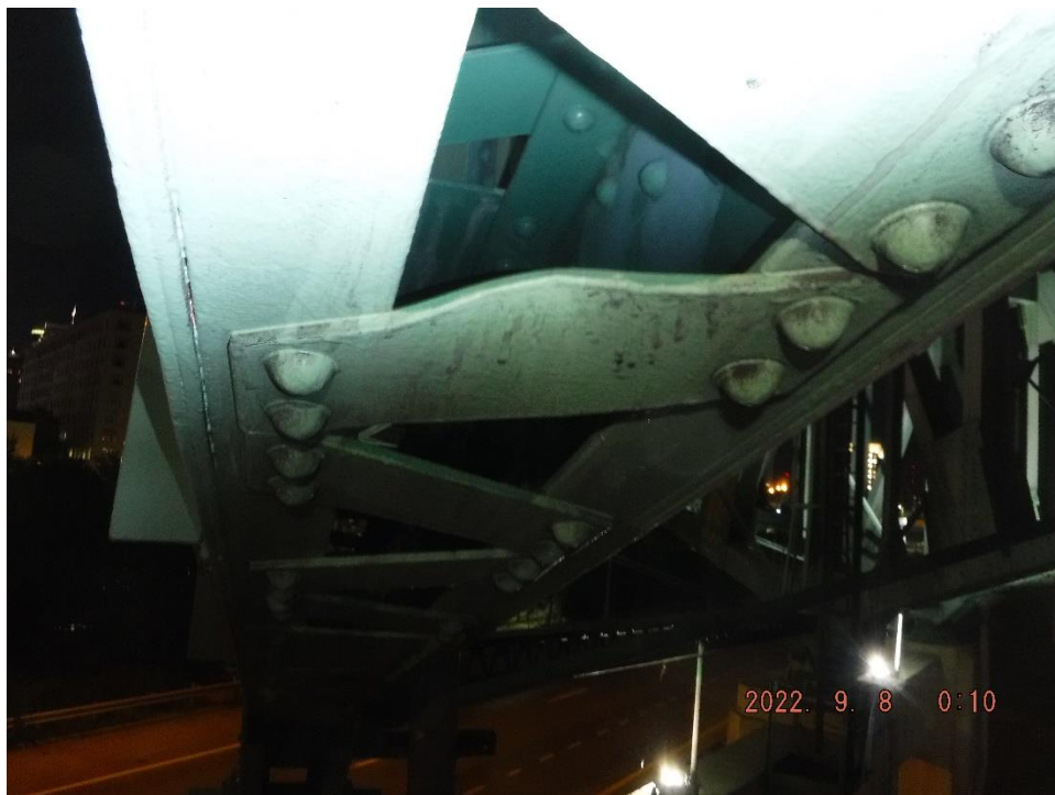
Photo 31: Bent lacing bar on L31-L32 in Span 9 of the South Truss
