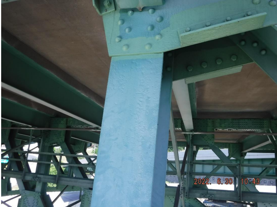
Photo 36: Painted-over pitting on the outside face of the member flange (South Truss, Span 10, L18-U18 shown)
