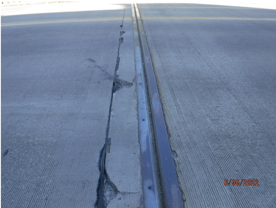
Photo 98: Spalls in the West Approach Slab at the expansion joint
