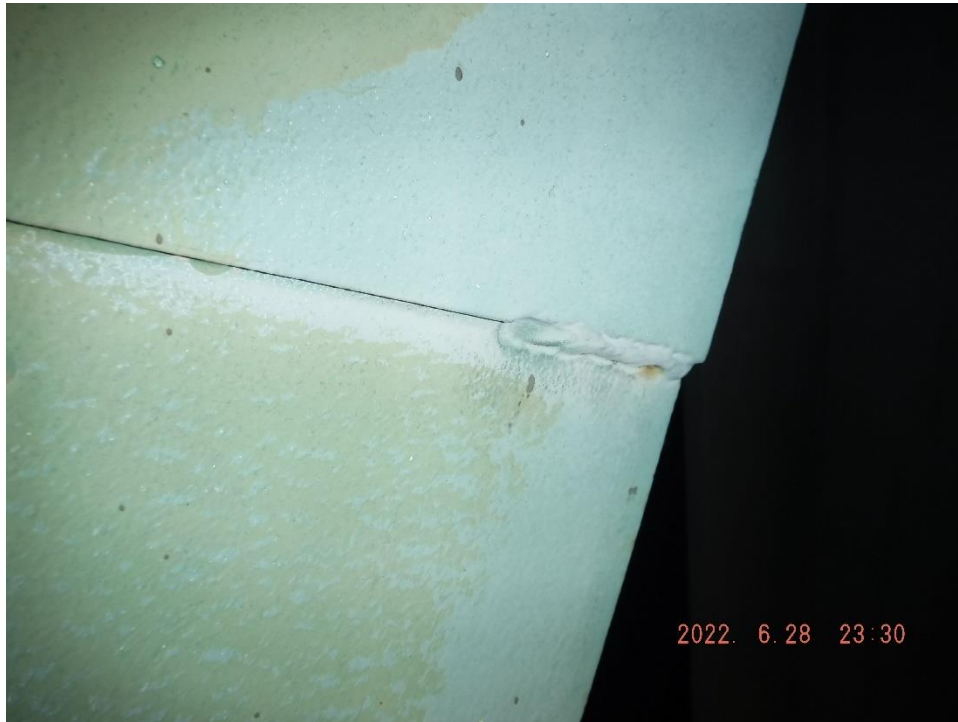
Photo 42: Undercut tack weld on fill plate (South Truss, Span 8, L29-U30 at U30 shown)
