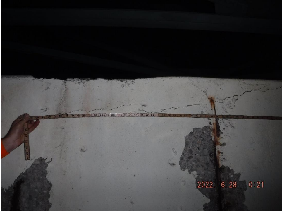
Photo 95: 4' long delamination on the east face of the Pier 13 Cap between the North and Center Columns
