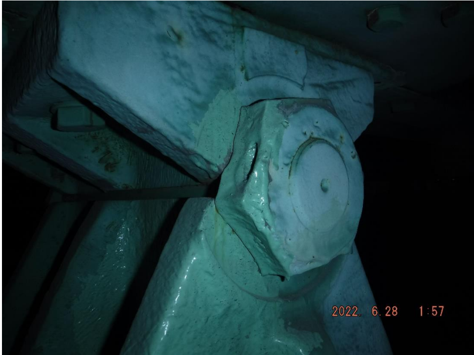
Photo 71: Gouge in pin nut at Pier 12, Center Girder, Span 12 Bearing
