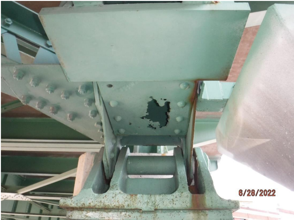
Photo 29: Example of corrosion hole and mis-drilled holes on batten plate (North Truss, Span 5, L0-L1 shown)
