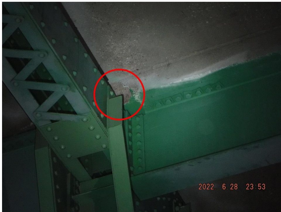
Photo 2: Example of an isolated haunch spall (South Truss, Span 8, North Face of U27 shown)
