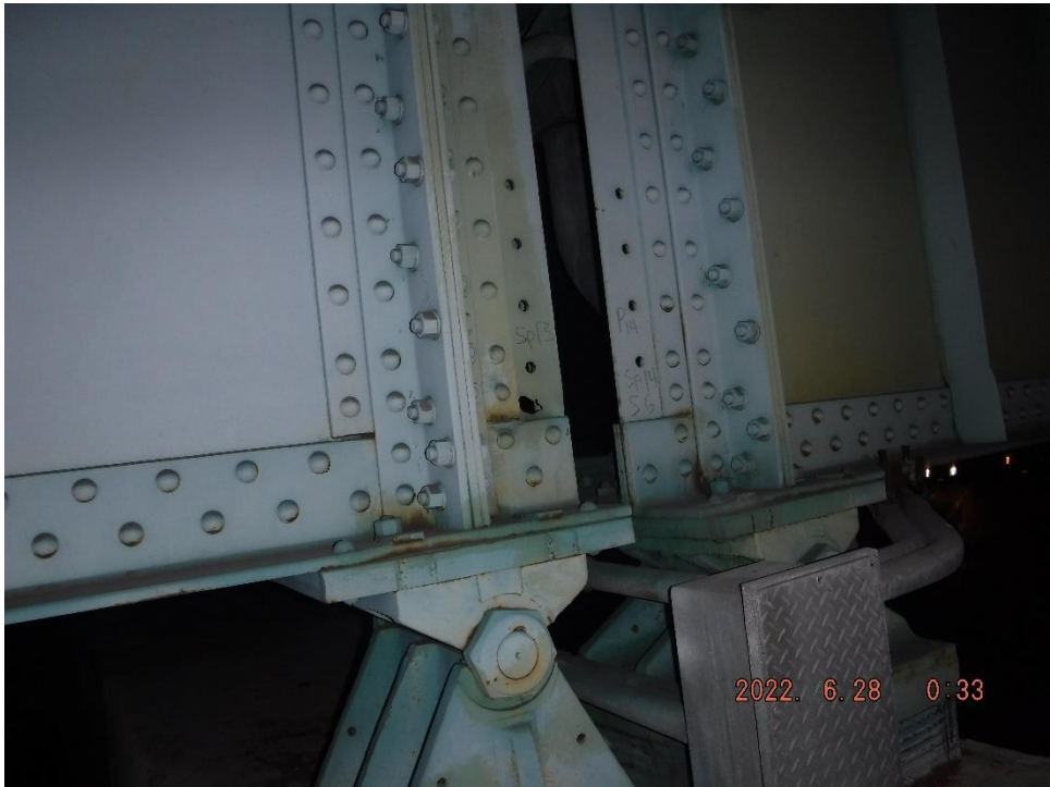
Photo 22: Example of mis-drilled holes (South Girder, Span 13 at Pier 14 shown)
