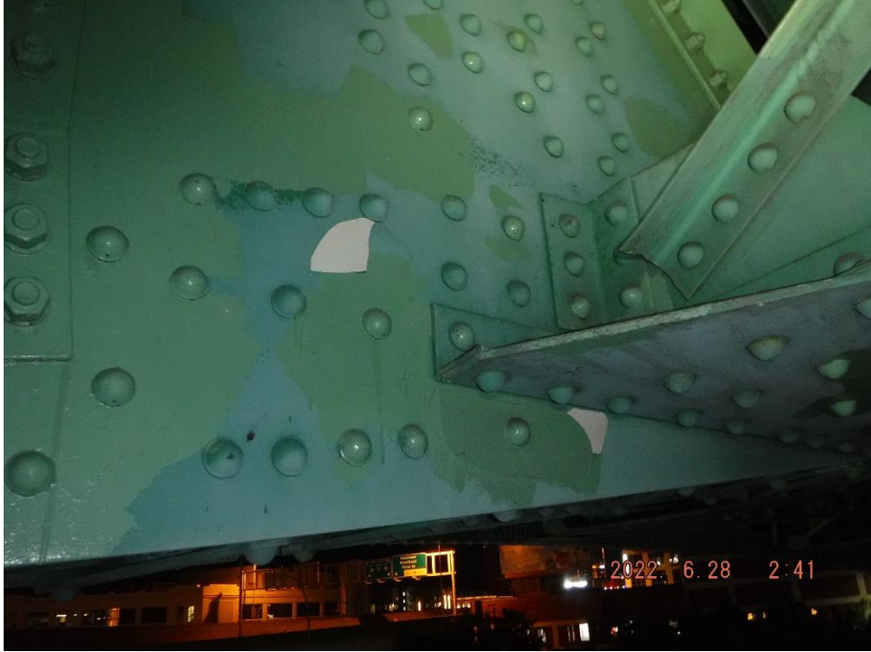
Photo 77: Chipped paint on gusset plate (Center Truss, Span 9, L42 shown)
