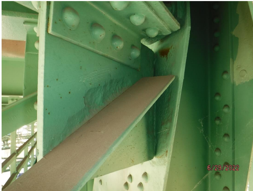
Photo 79: Painted-over pitting on connection plate (Center Truss, Span 7, U0 shown)
