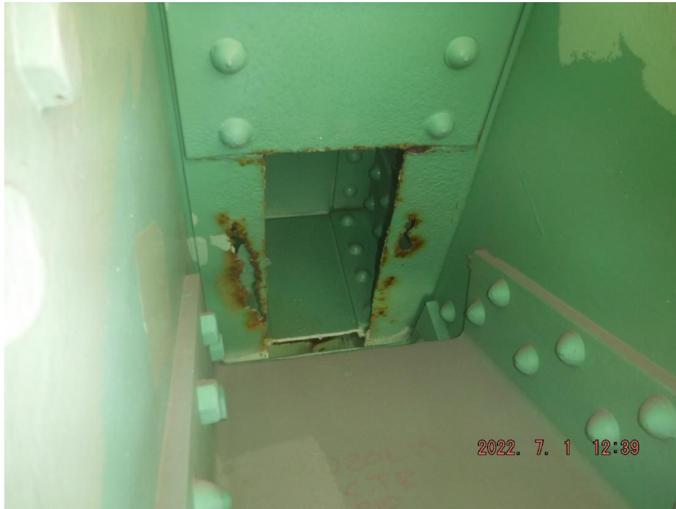
Photo 32: Example of reactivating corrosion hole on member top flange (South Truss, Span 10, U20 shown)
