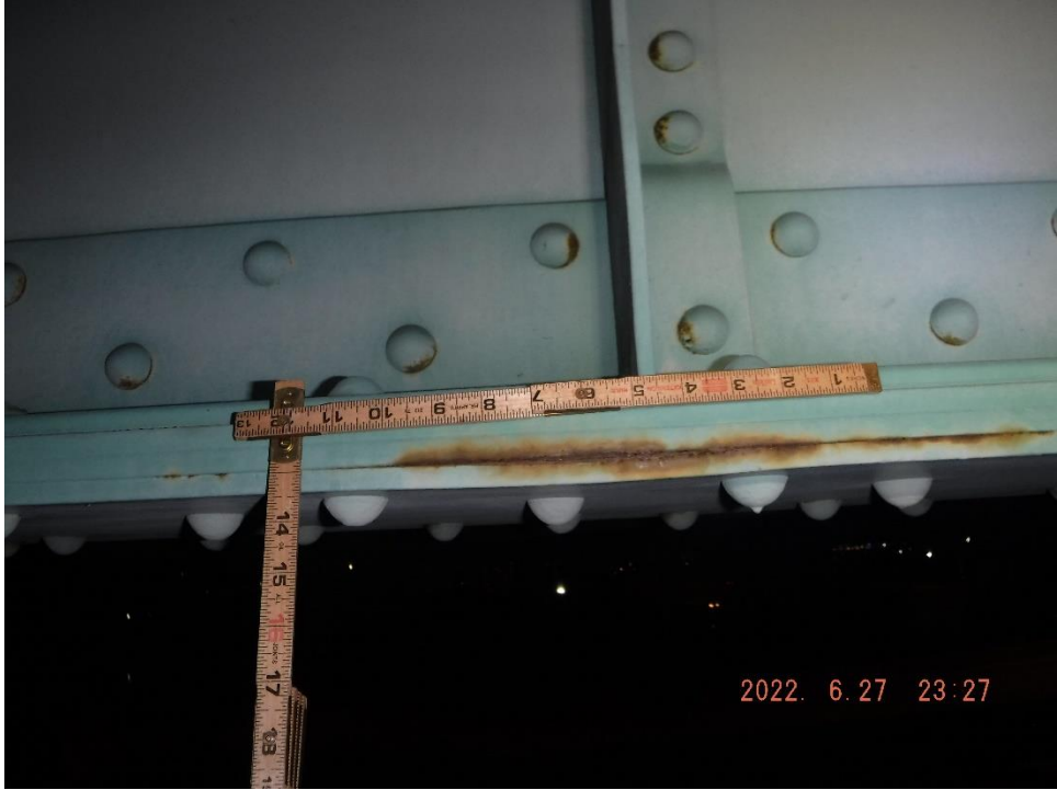
Photo 21: Example of active pack rust between flange plates (North Girder, Span 14 near midspan shown)
