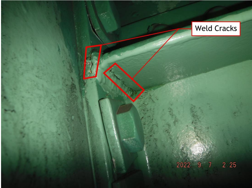
Photo 41: Cracked weld on web stiffener at U37 on member U37-L37
