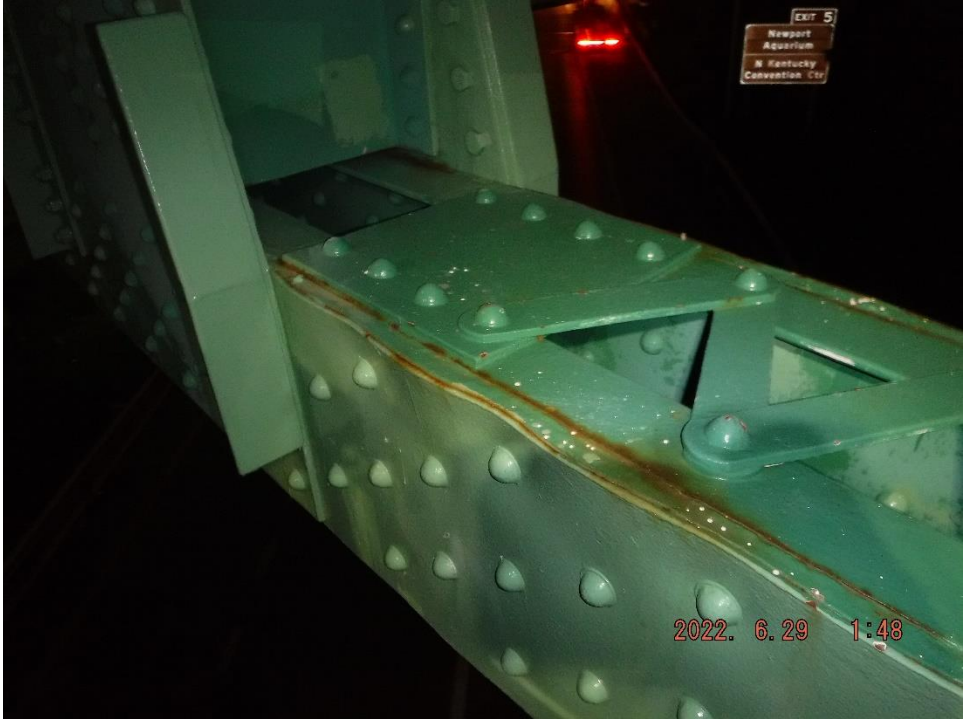
Photo 26: Example of widespread pack rust and out of plane plate bending (North Truss, Span 8, L28-L29 Web shown)
