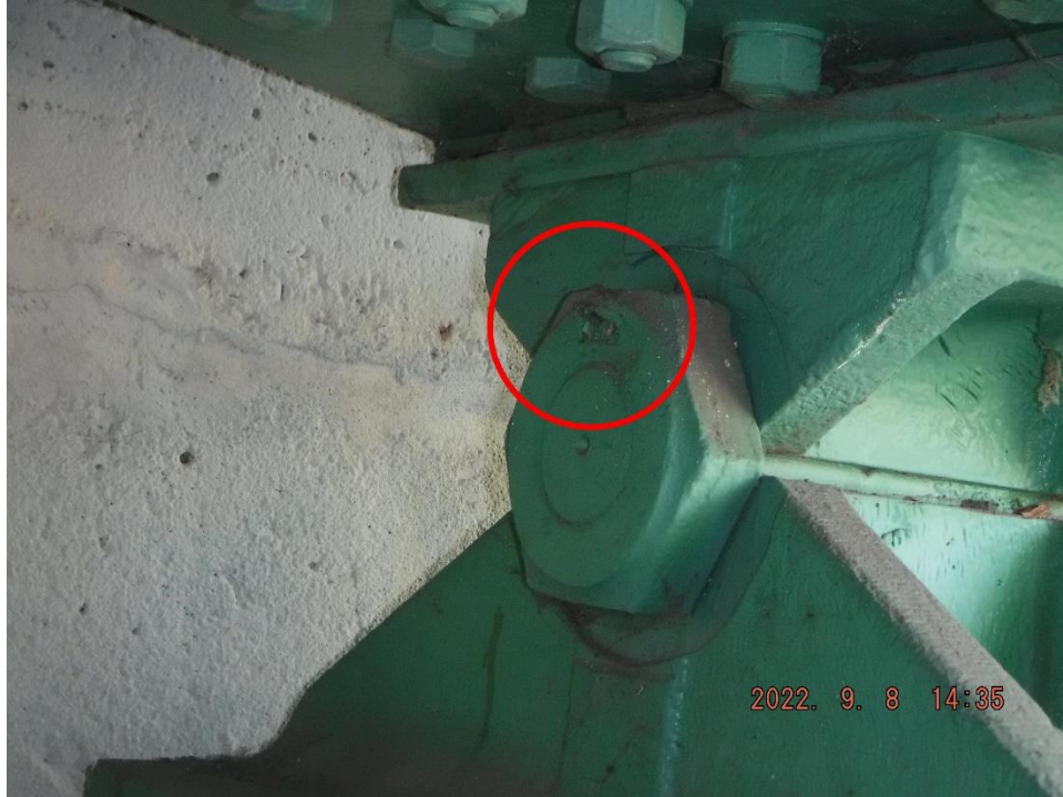
Photo 74: Manufacturing defect on the North Bearing at the West Abutment
