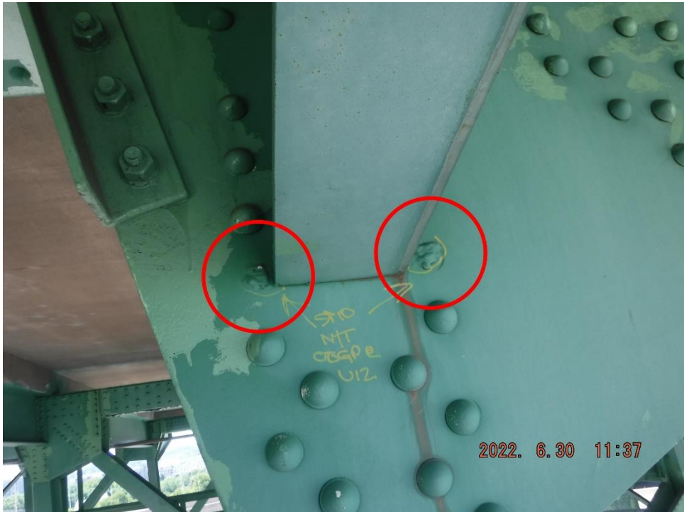
Photo 59: Mis-drilled holes that have been filled with plug welds (Span 10, North Truss, U12, North Gusset shown)
