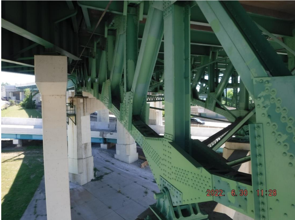
Photo 76: Typical paint condition on truss (North Truss, Span 10 shown)
