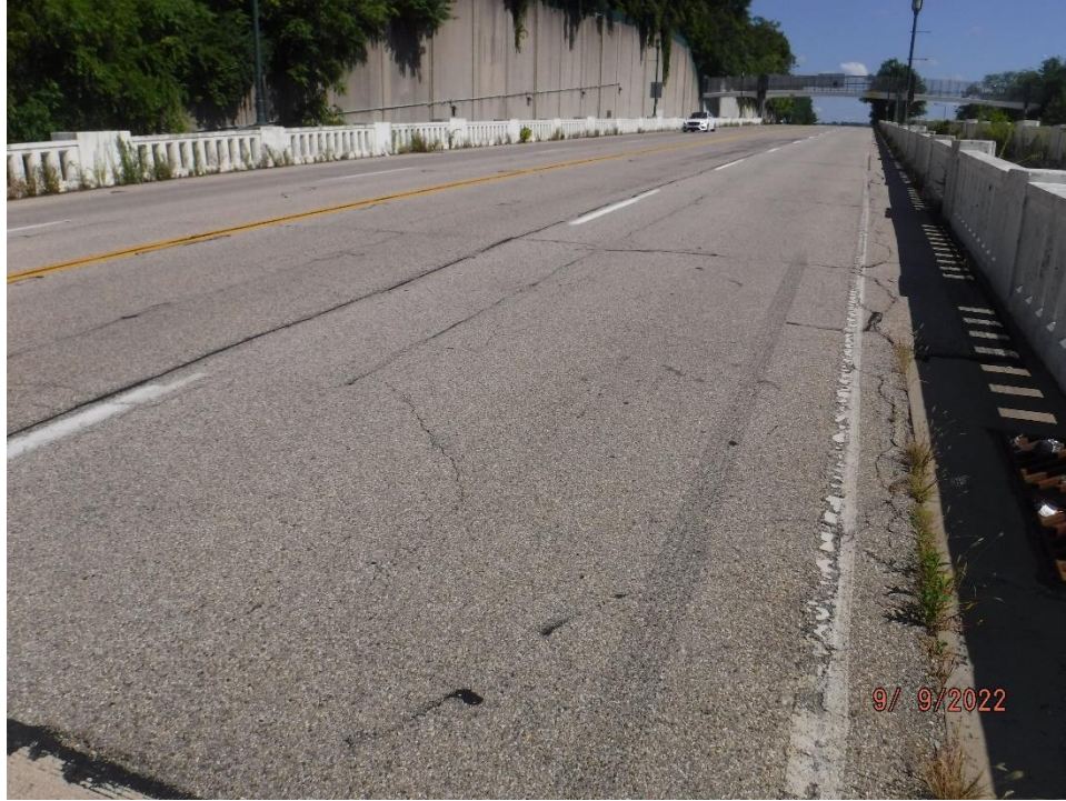
Photo 100: East approach pavement with unsealed cracks in the travel lanes and near the south edge
