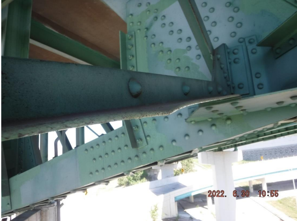
Photo 80: Bent cross brace member in Span 10 between L18 on the Center Truss and L20 on the North Truss
