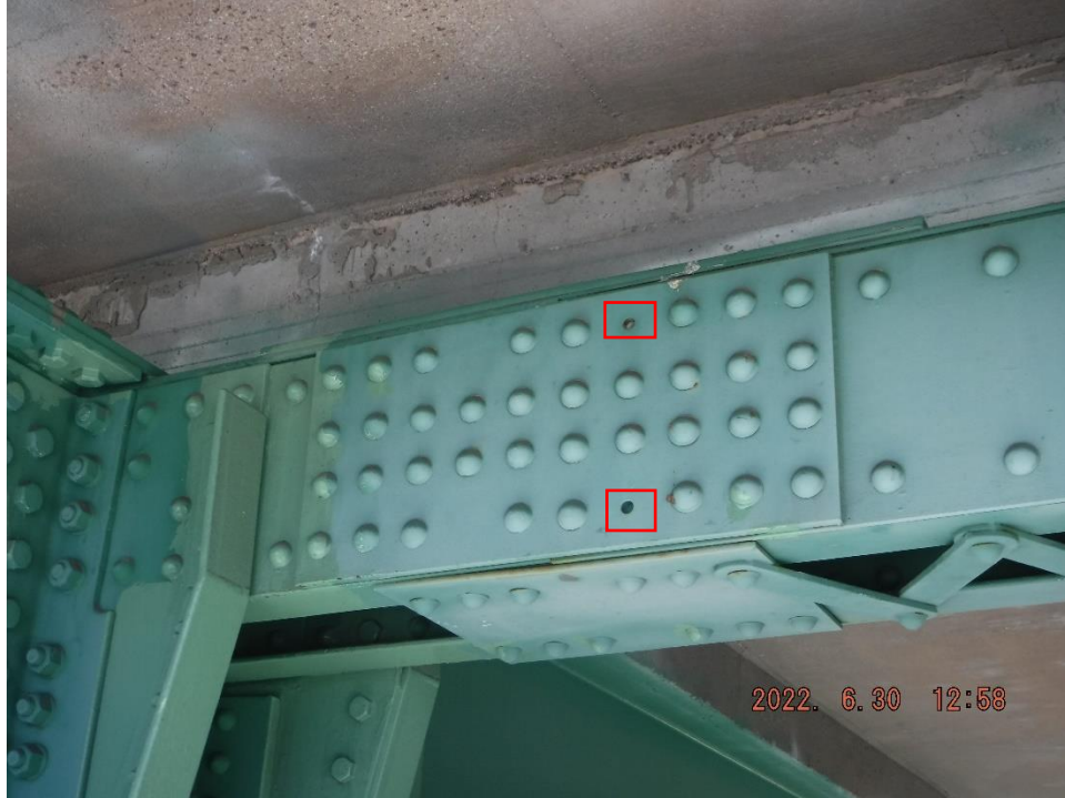
Photo 35: Example of mis-drilled holes and bent cover plate due to missing fill plate (South Truss, Span 10, U10-U11 shown)
