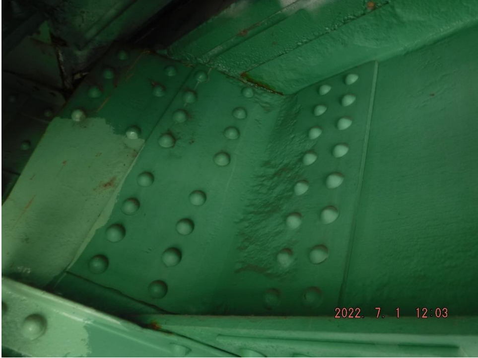
Photo 46: Painted-over section loss in connection plate and top flange (Center Truss, Span 10, South Bay at U20 shown)
