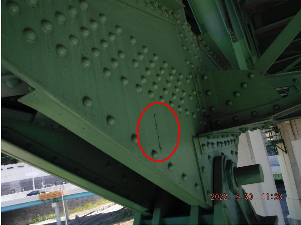
Photo 58: Gouge in gusset plate where attachment was previously welded (Span 10, North Truss, L8, South Gusset shown)
