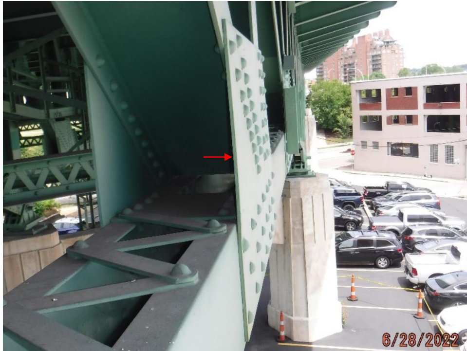
Photo 66: Minor free edge bowing without pack rust at unrepaired gusset edge (Span 5, South Truss, L3, South Gusset shown)
