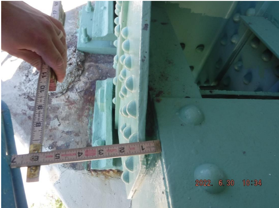
Photo 64: Free edge localized deformation with pack rust at unrepaired gusset edge (Span 10, South Truss, L20, South Gusset shown)
