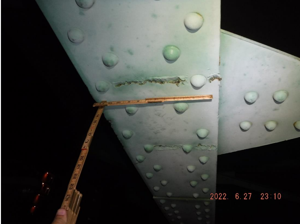
Photo 19: Flame cut gouge on bottom flange of girder (North Girder, Span 15 near Pier 15 shown)
