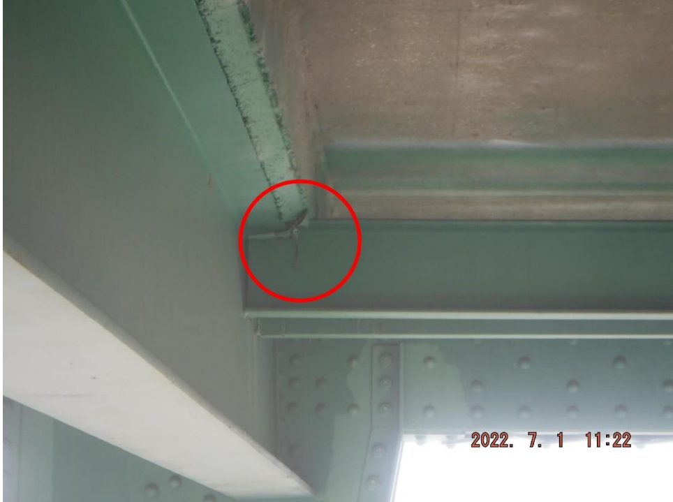
Photo 16: Cracked drainage support channel at the south end of Pier 9
