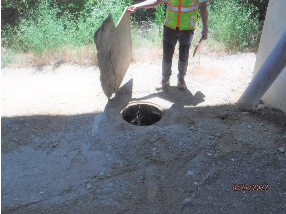
Photo 17: Open manhole covered with plywood, East of Column 3 at Pier 15
