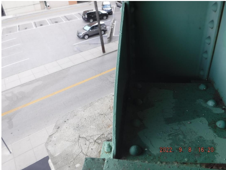
Photo 65: Free edge bowing with pack rust at unrepaired gusset edge (Span 5, South Truss, L0, South Gusset shown)
