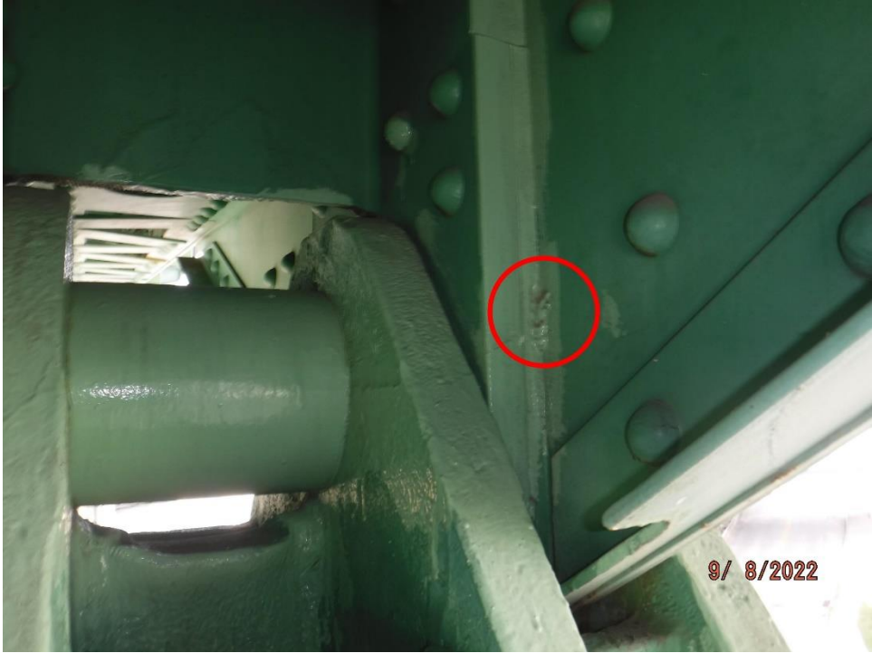
Photo 72: Undercut tack weld between gusset plate and pin plate (Span 11, Center Truss, L8 at Pier 11 shown)
