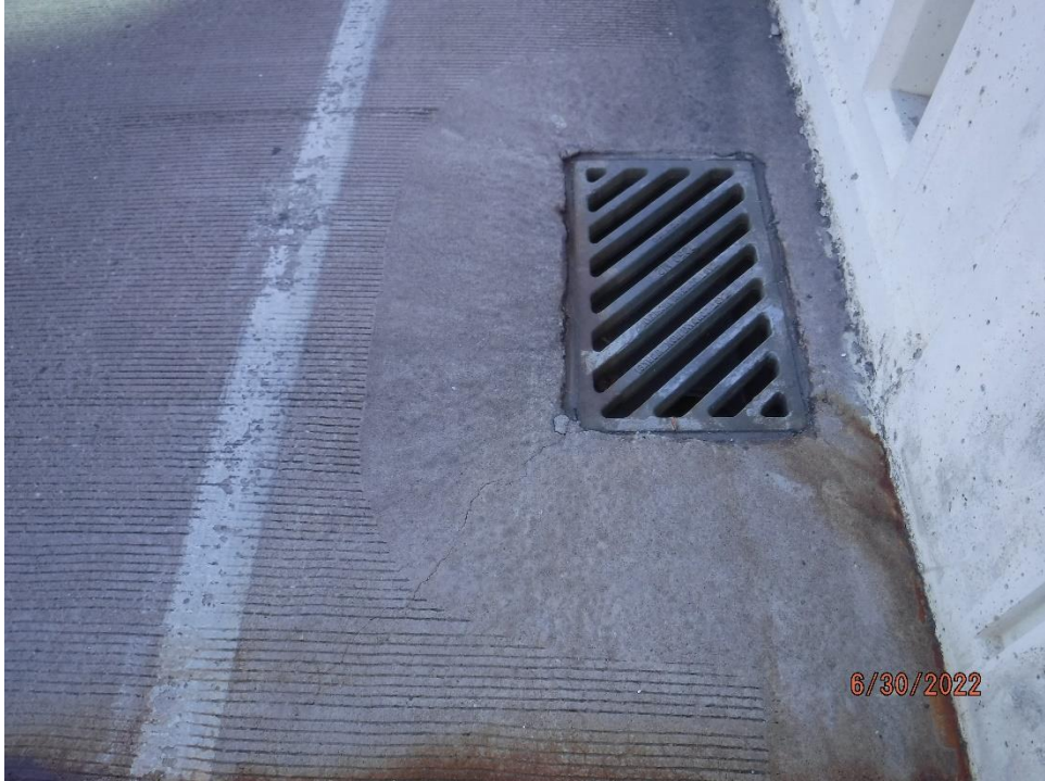
Photo 6: Typical radial cracks at drainage grate
