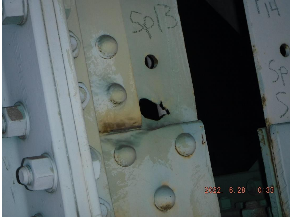
Photo 25: Corrosion hole in the web on South Girder, Span 13 at Pier 14
