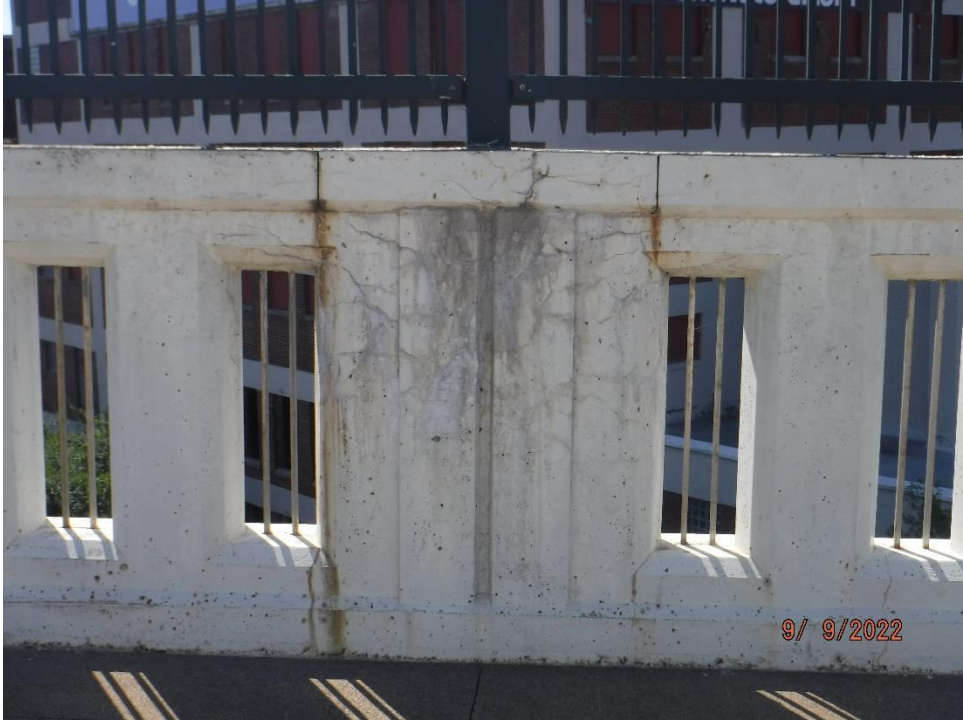
Photo 11: Cracking and rust staining on interior face of bridge railing (South Railing Span 7 shown)
