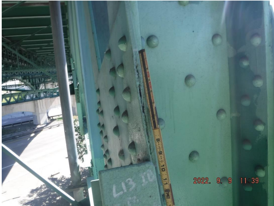
Photo 60: Laminar tear in the North Gusset Plate at L13 in Span 7 of the South Truss
