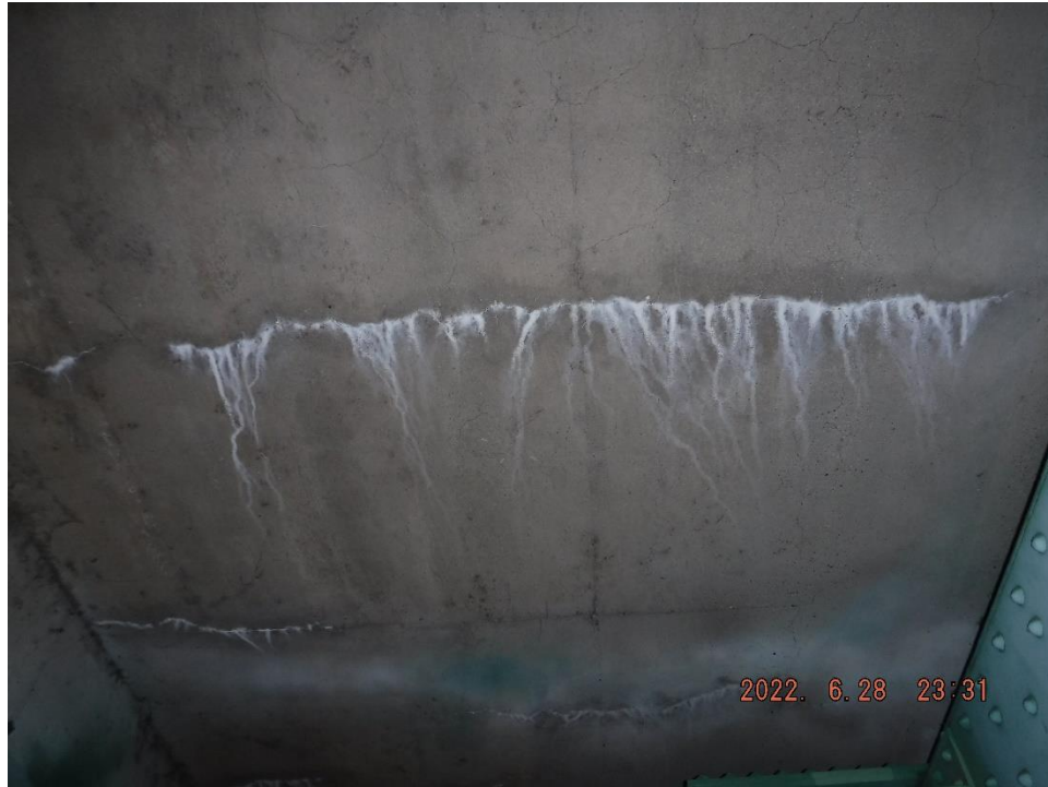
Photo 1: Typical transverse and map cracking between cantilever overhang brackets (South overhang, Span 8, between U29 and U30 shown)
