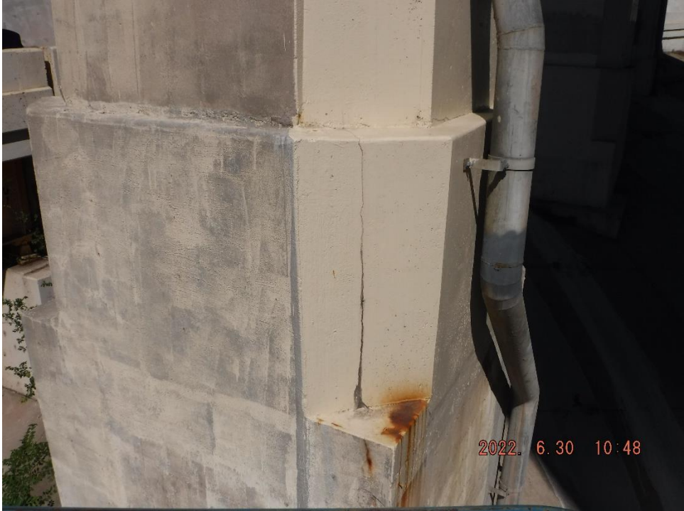
Photo 82: Vertical crack in the South Column of Pier 10
