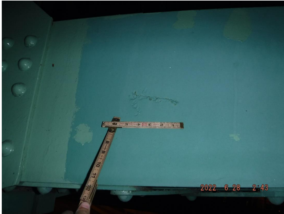
Photo 30: Example of gouge in member web (Center Truss, Span 9, L42-L44 shown)
