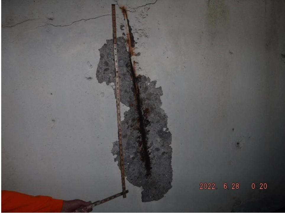
Photo 94: 3' x 1' spall with exposed reinforcement on the east face of the Pier 13 Cap between the North and Center Columns
