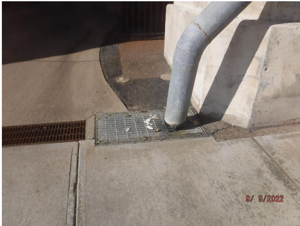
Photo 13: Example of debris in drainage grate at ground termination (Column 3 of Pier 3 shown)
