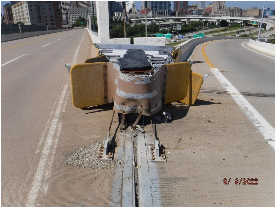
Photo 12: Example of impact attenuator damage (East Attenuator shown)
