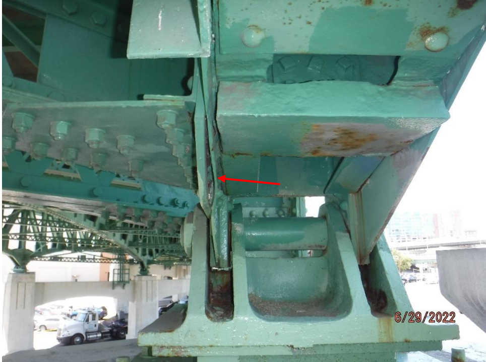
Photo 61: Section loss on gusset plate and bowing due to pack rust at bearing connection (Span 7, North Truss, L0, South Gusset shown)
