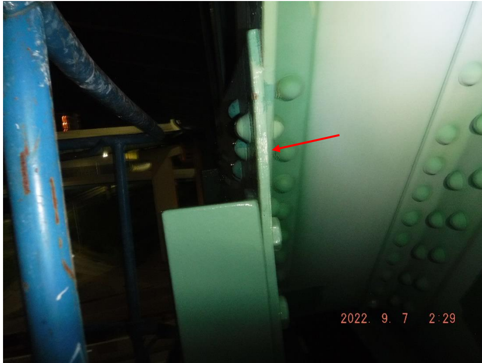
Photo 67: Free edge bowing at repaired gusset edge (Span 9, North Truss, L37, North Gusset shown)
