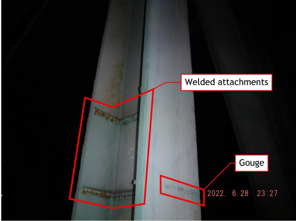
Photo 40: Welded attachment remains and gouge in member flange (South Truss, Span 8, L30-U30 shown)
