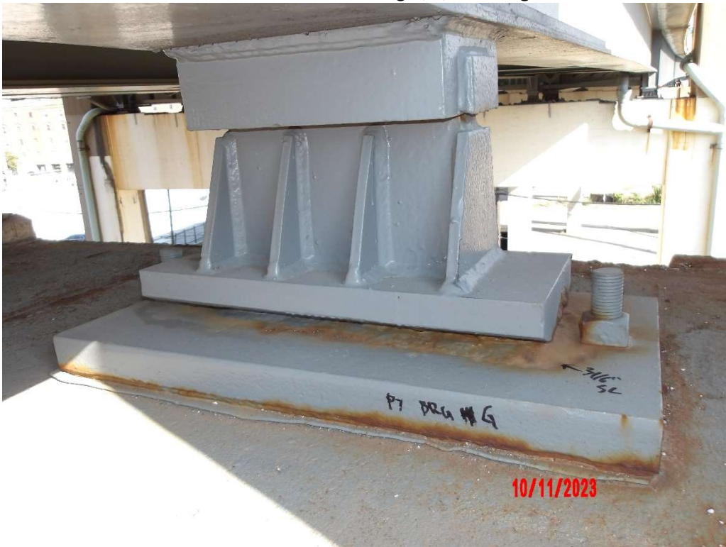
Photo 52- Pier 7 Bearing G, 3/16" Section Loss Masonry Plate
