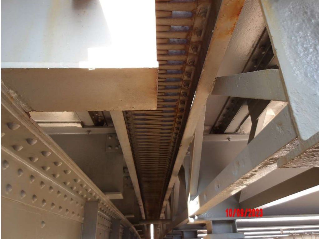
Photo 16- Truss Finger Joint at Pier 0
