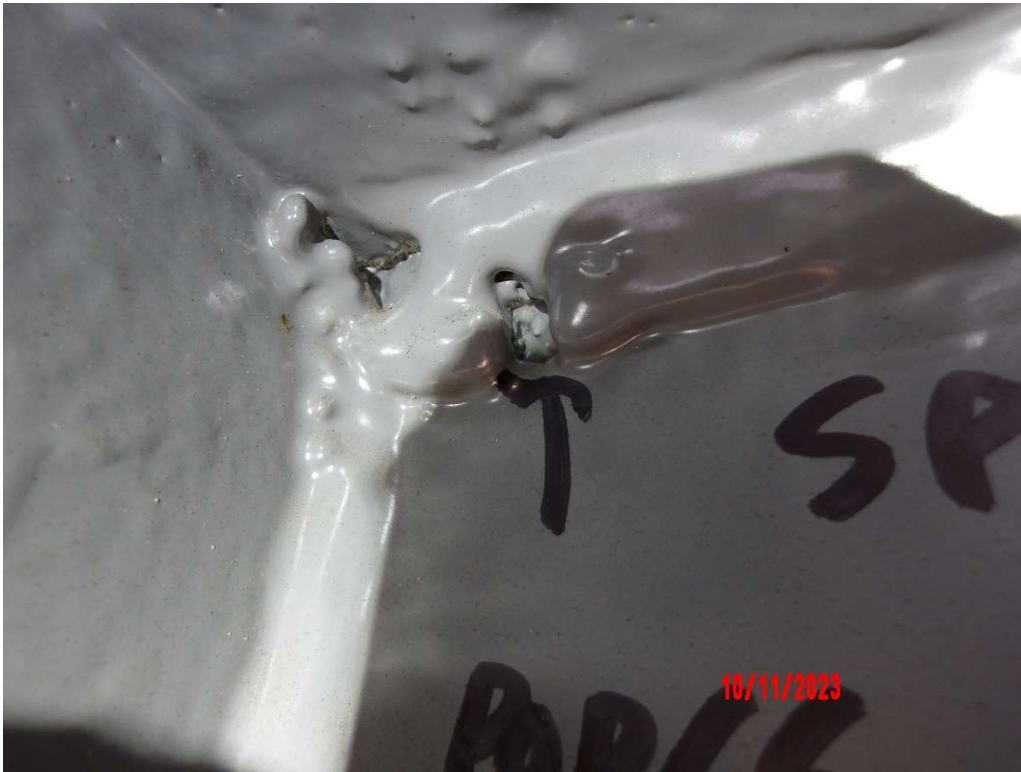
Photo 42- Girder D, Span 12, Pores
