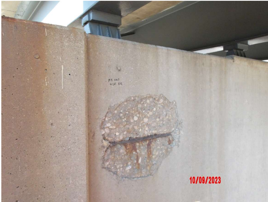
Photo 89- Pier 3, Column 2, 4 SF Spall with Exposed Rebar
