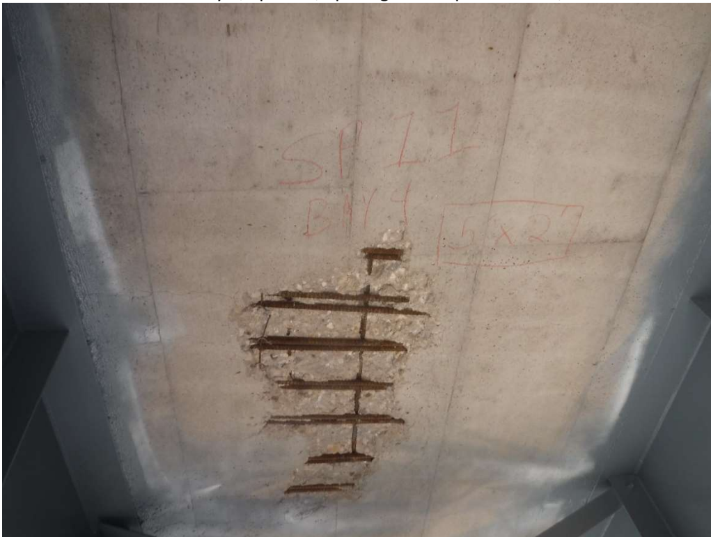
Photo 2- Span 11, Bay 4, 10SF Spall with Exposed Rebar
