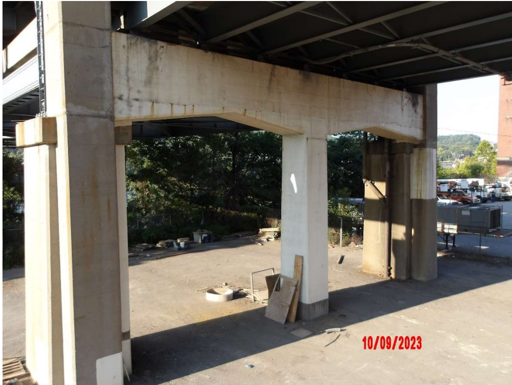
Photo 80- Pier 0, Front Face, FRP Wrap Delaminations and Staining
