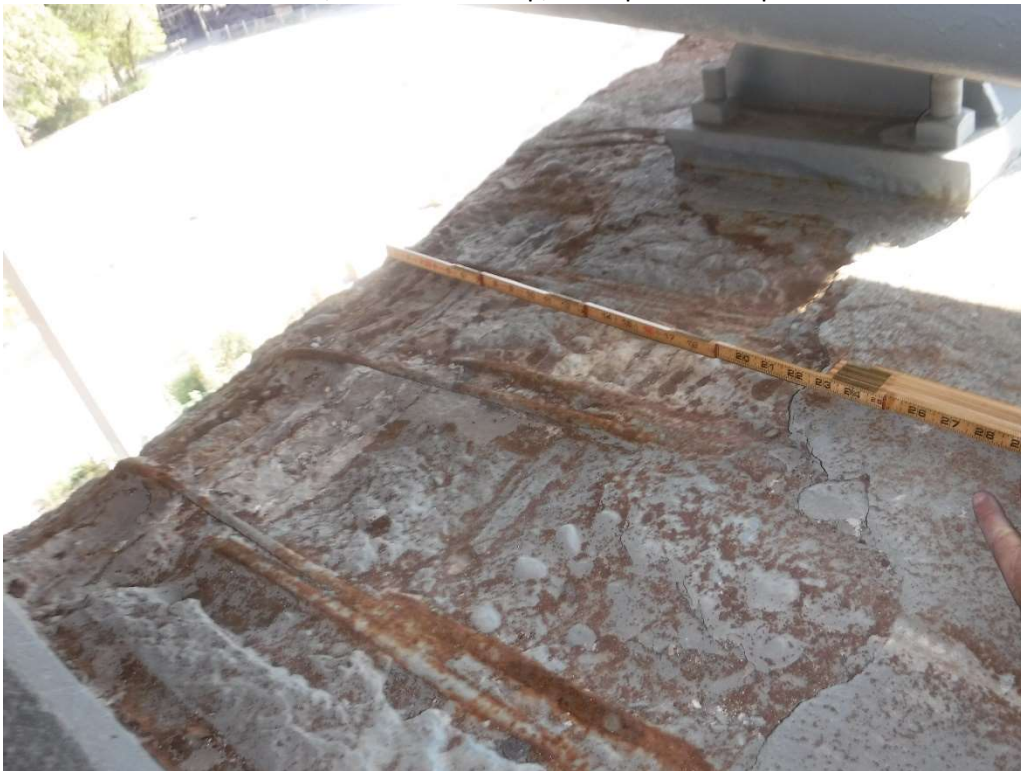
Photo 94- Pier 11, Top Cap, Near Girder H, Spalling with Exposed Rebar 14SF
