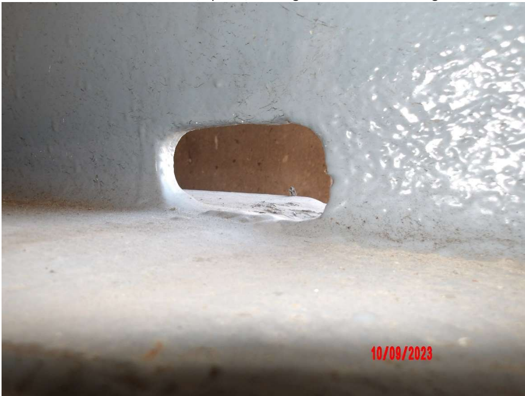
Photo 29- Girder A, Web, Hole, Near Pier 0
