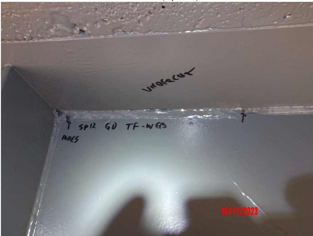
Photo 43- Girder D, Span 12, Undercut Weld and Pores
