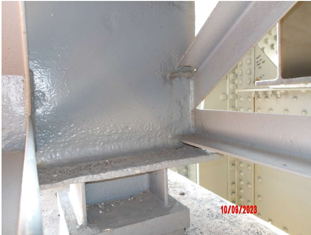
Photo 62- Cross Frames, Pier 0, Typical Section Loss
