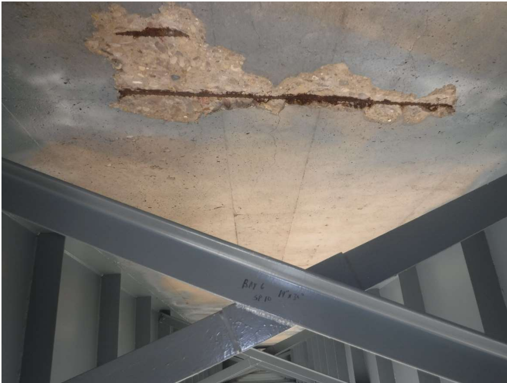
Photo 1- Bay 6, Span 10, Spalling with Exposed Rebar, 6SF
