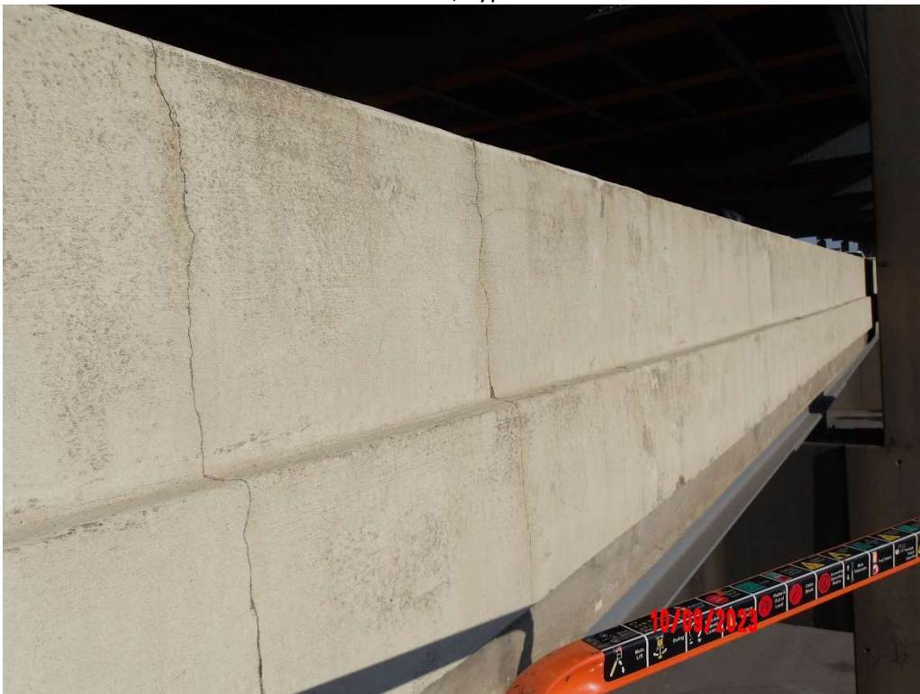
Photo 20- Typical Barrier Cracking
