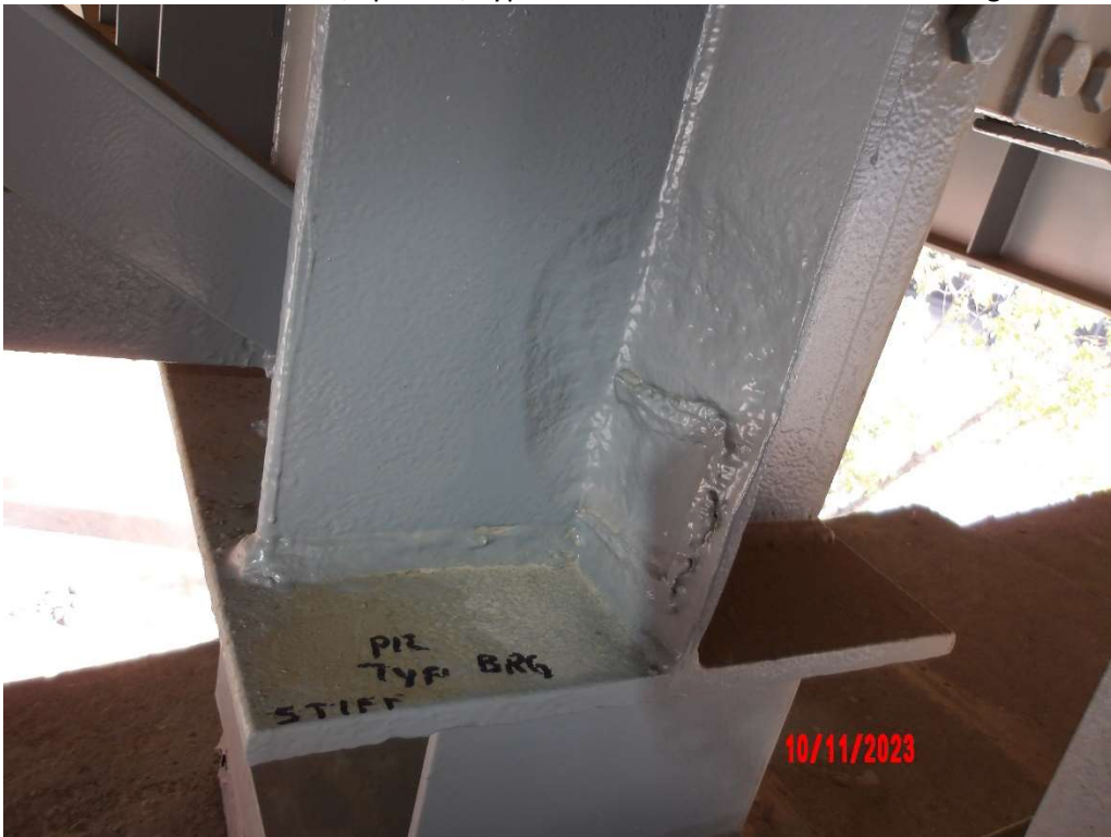
Photo 41- Girder D, Span 12 at Pier 12 OB, Weld Remnants
