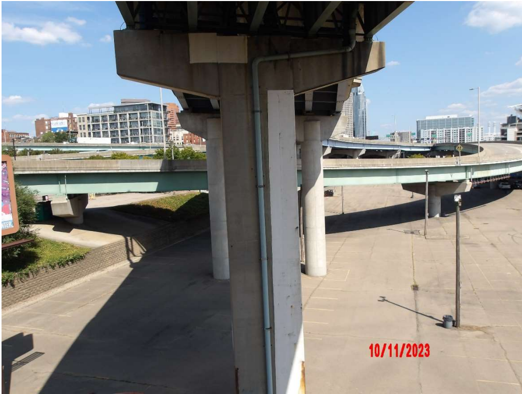
Photo 84- Pier 20D Back Face, Note FRP Wrap Delaminations
