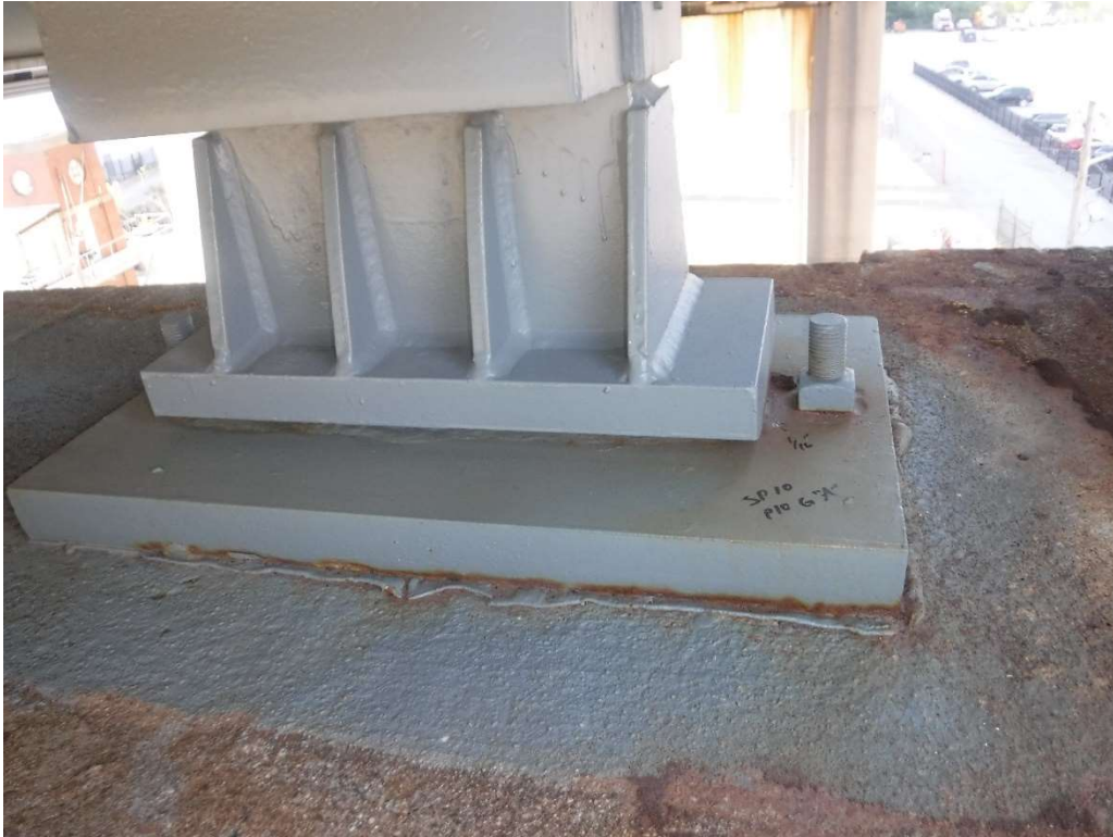
Photo 53- Pier 10, Bearing A, 1/16" Pitting Underneath
