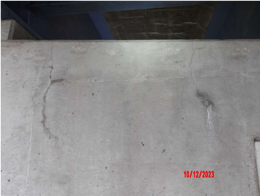
Photo 95- Pier 2C, Vertical Cracking 2' L at 2' Spacing
