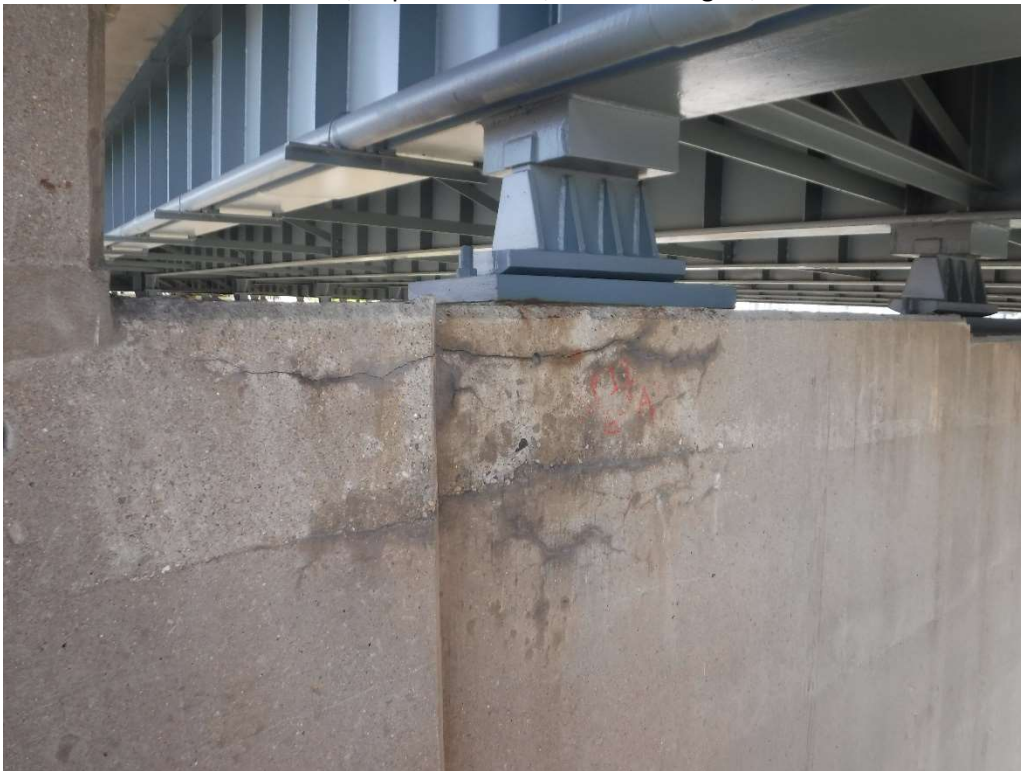
Photo 92- Pier 11, Girder A, Delamination 8 SF
