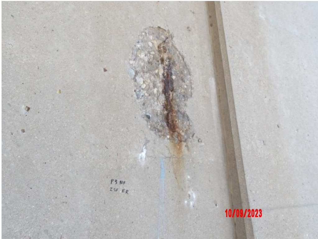
Photo 87- Pier 3, North Face Cap, 2 SF Spall with Exposed Rebar
