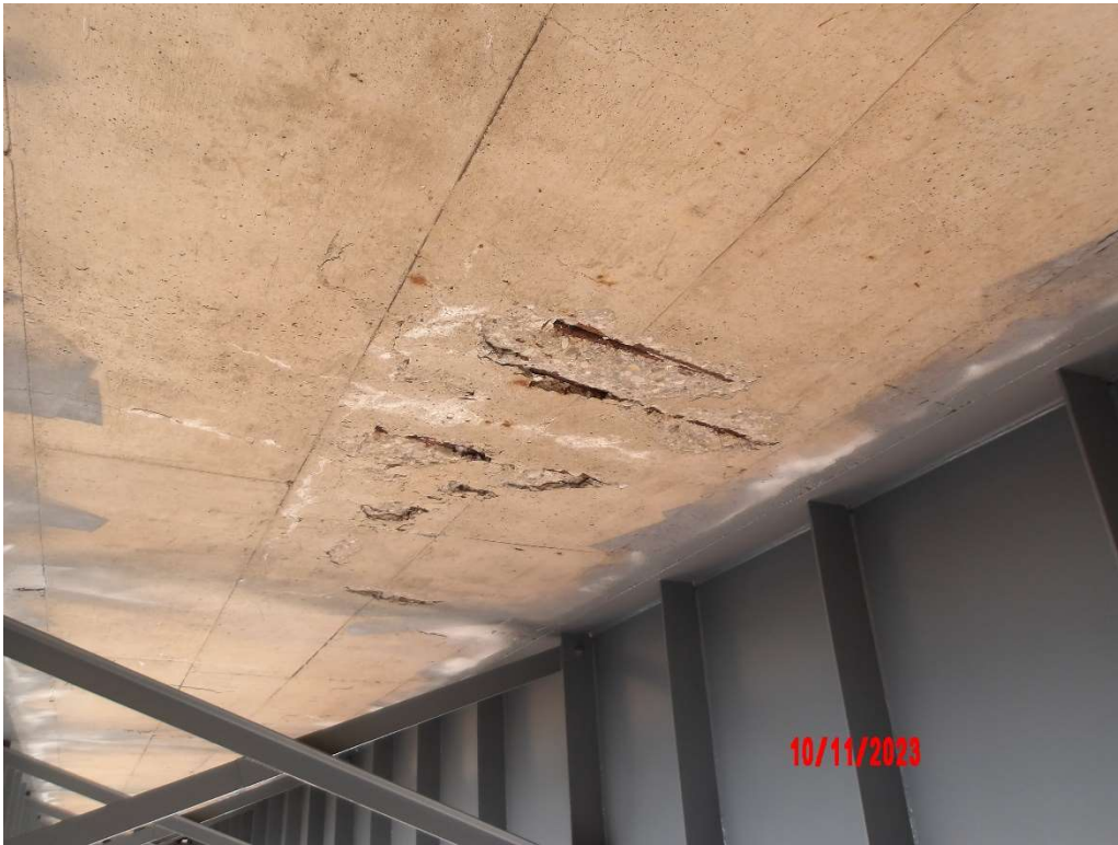
Photo 3- Span 12, Bay 4, 15 SF Spalling with Exposed Rebar
