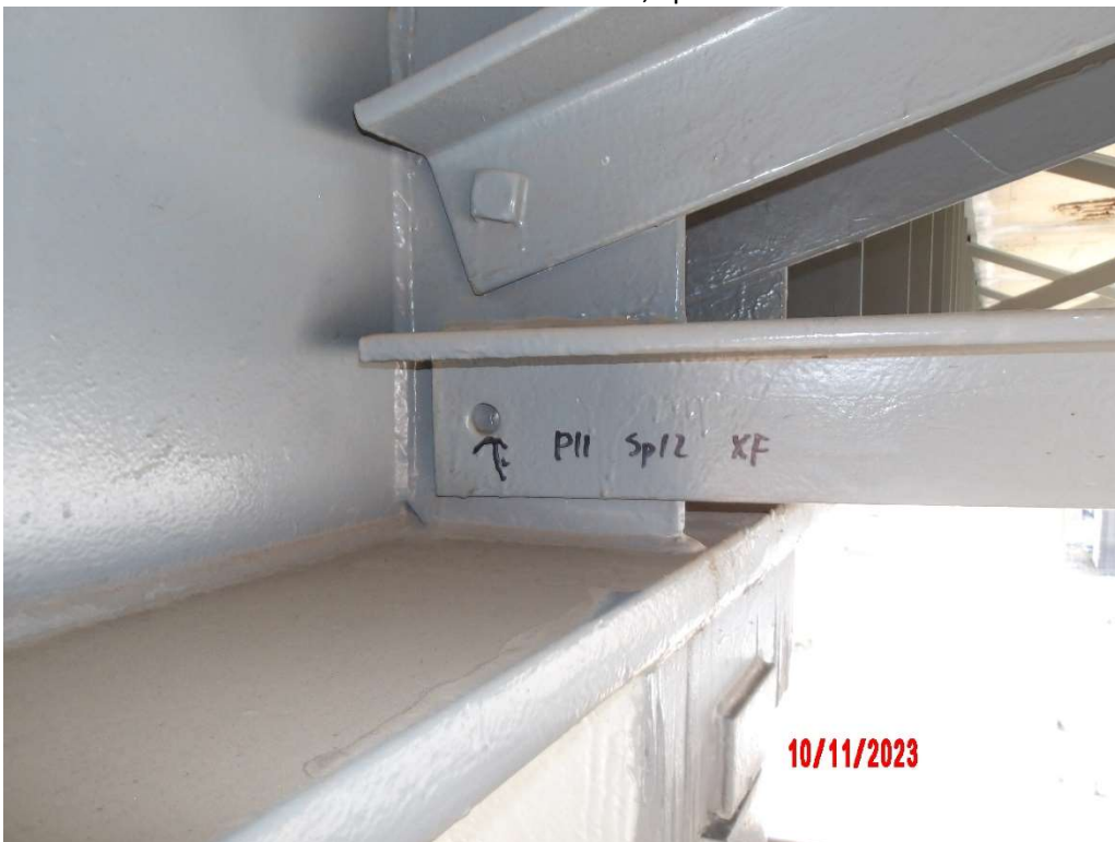
Photo 64- Cross Frame, Pier 11, Span 12, Typical Welded Details, Missing Bolts
