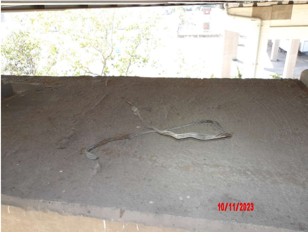
Photo 96- Disconnected Ground Wire on Pier 13
