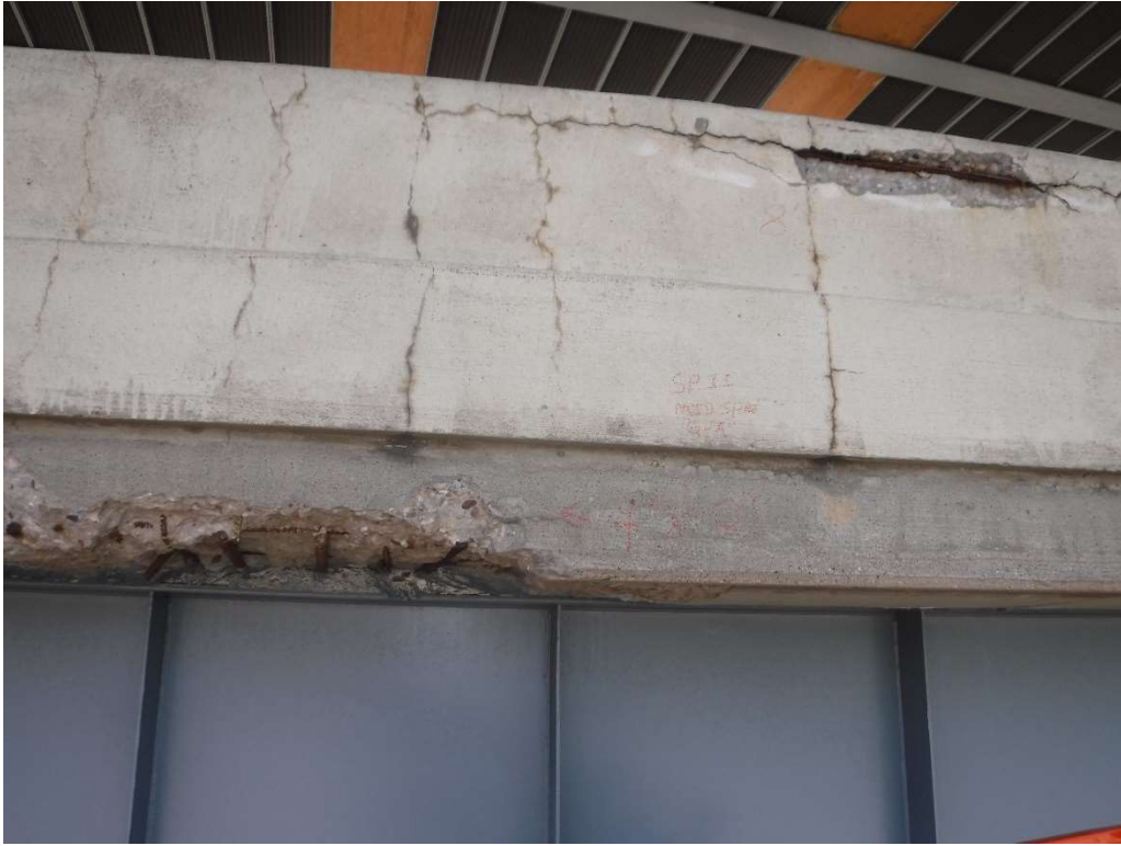
Photo 21- Span 10, Barrier, Typical Spalling and Cracking
