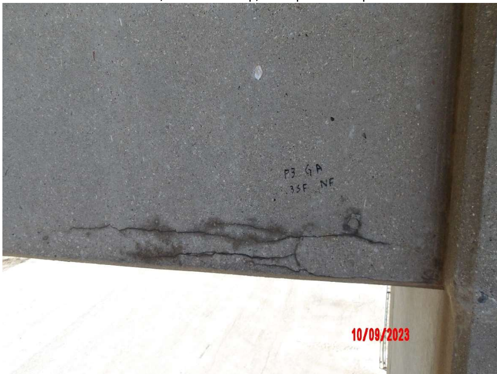
Photo 88- Pier 3, North Face Cap, 3 SF Delamination
