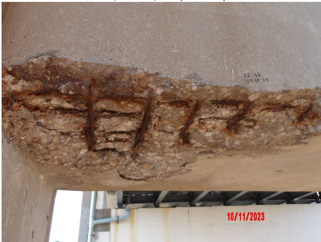
Photo 90- Pier 5 Cap at Column 2, 12 SF Spall with Exposed Rebar
