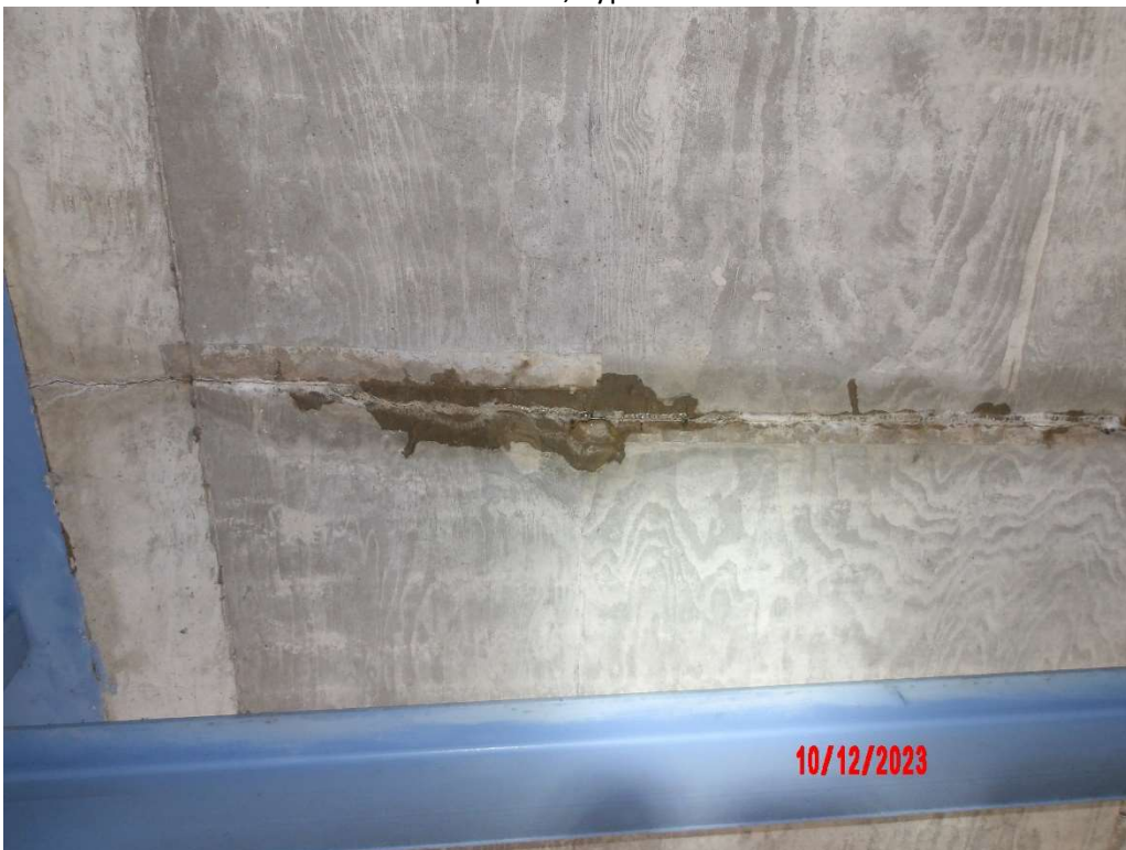
Photo 12- Span 23, Transverse Crack, Leaking Water
