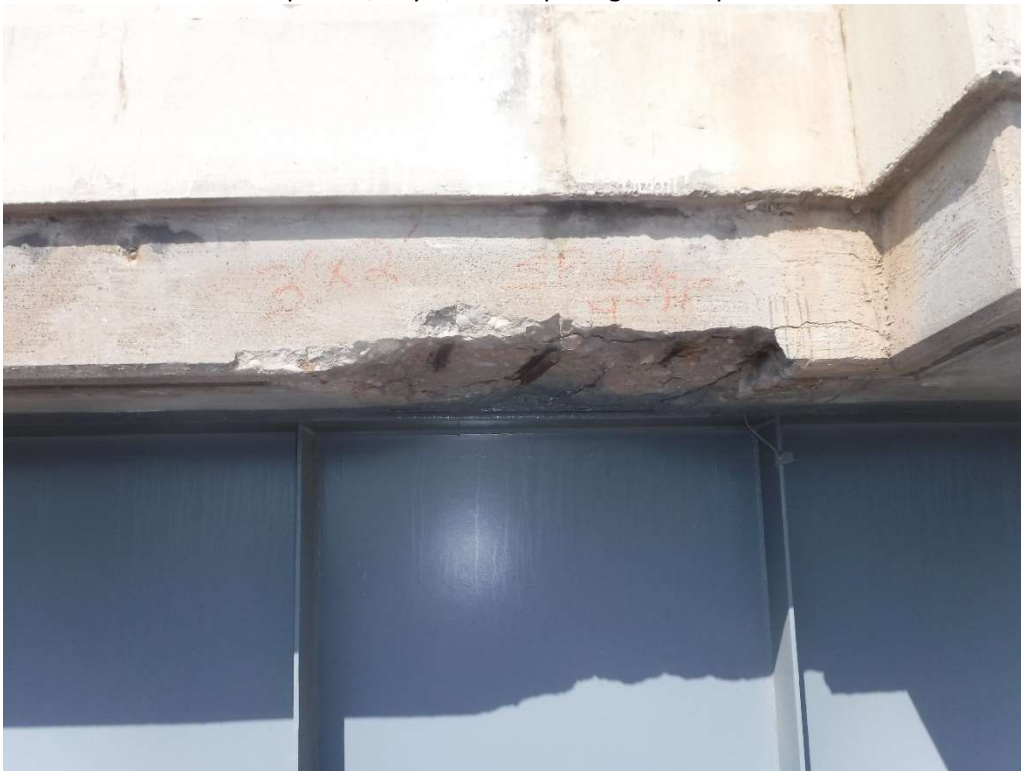
Photo 4- Span 12, Overhang, 6SF Spall with Exposed Rebar
