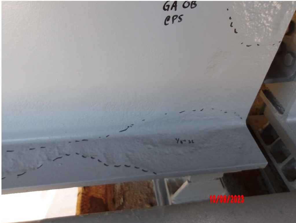
Photo 34- Girder A, Bottom Flange at Pier 5, Section Loss 1/8" Web
