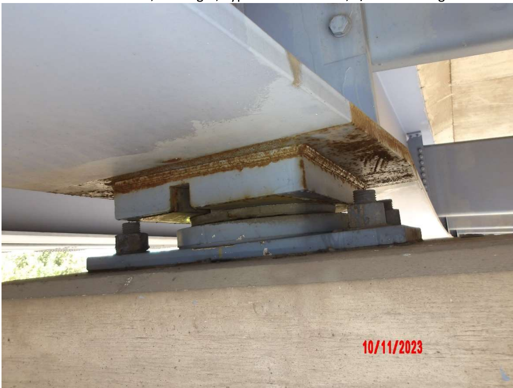
Photo 61- Pier 1C, Bearings Typical Freckled Rust
