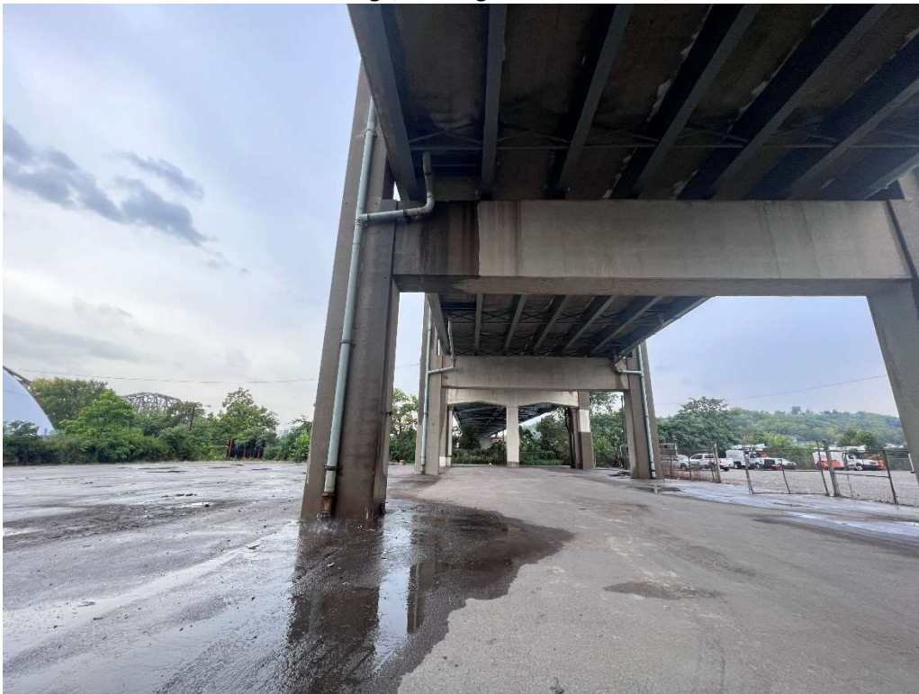
Photo 24- Drainage, Leaking on Substructure, Pier 3
