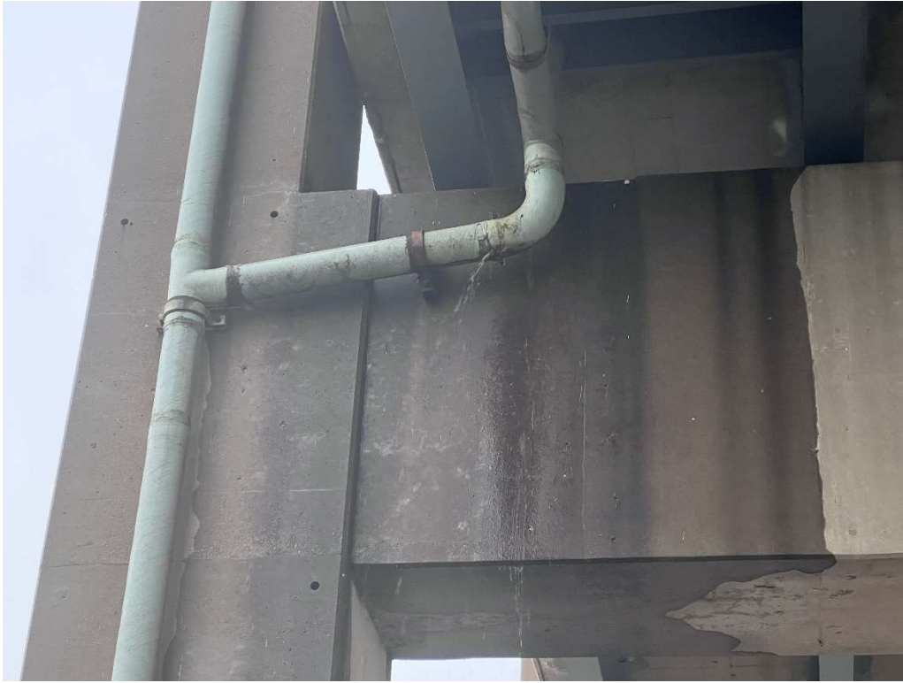
Photo 23- Drainage, Leaking on Substructure, Pier 3
