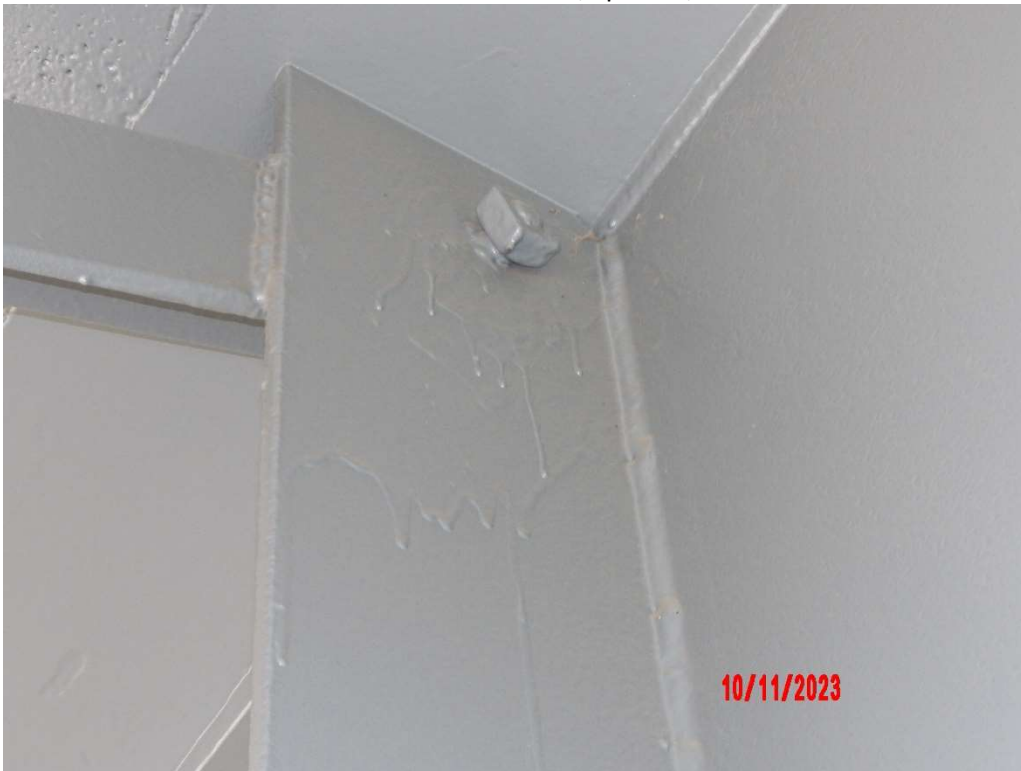
Photo 68- Cross Frame Loose Connection, Bay 6, Span 14
