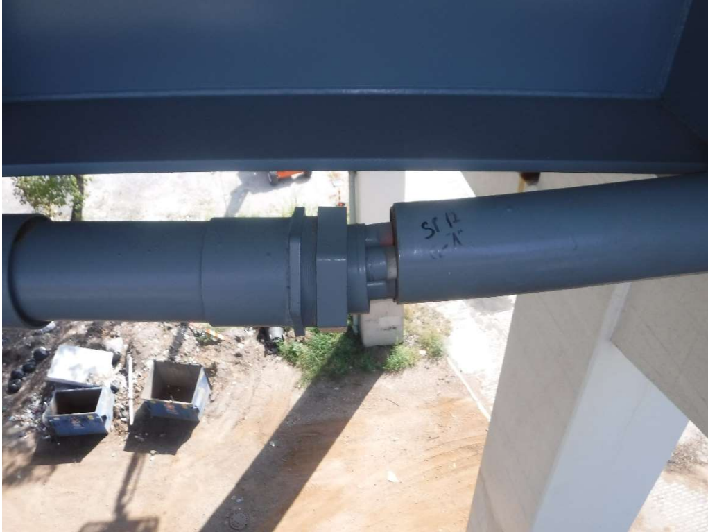
Photo 99- Span 12, Conduit Broken under Girder A
