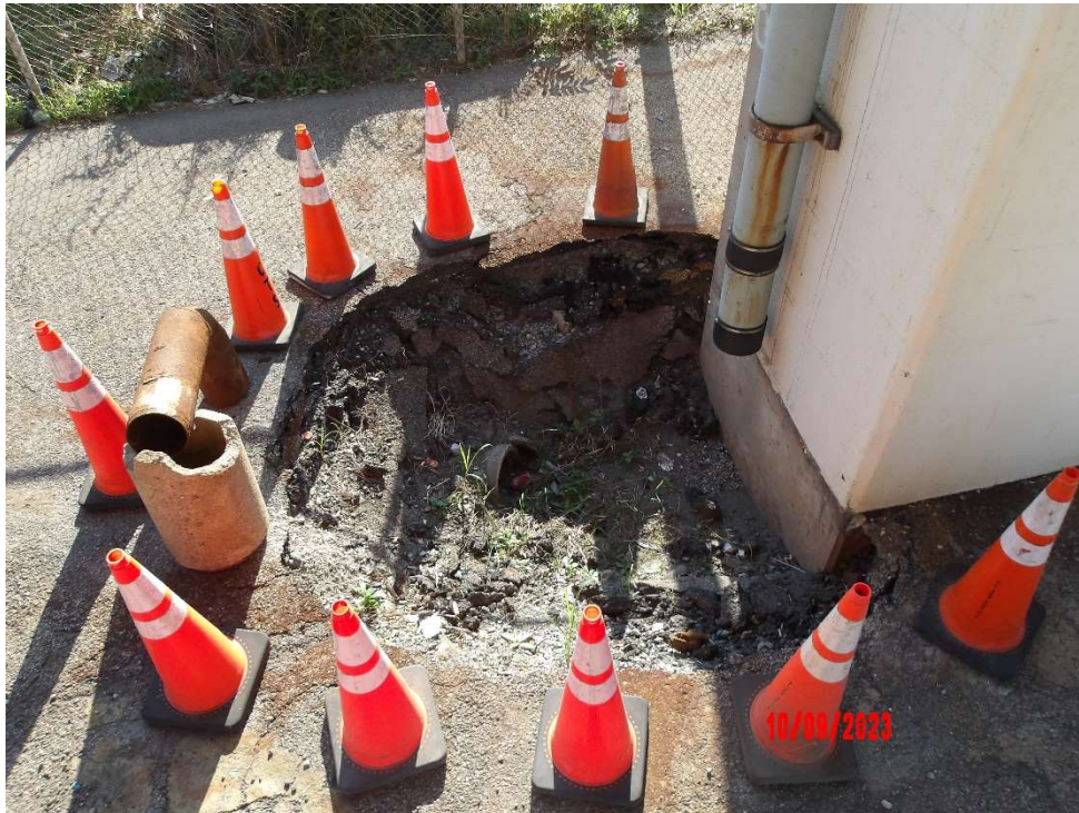
Photo 25- Pier 4, Column 2, Drain Failure with 8' Diameter Erosion Hole up to 4' Deep
