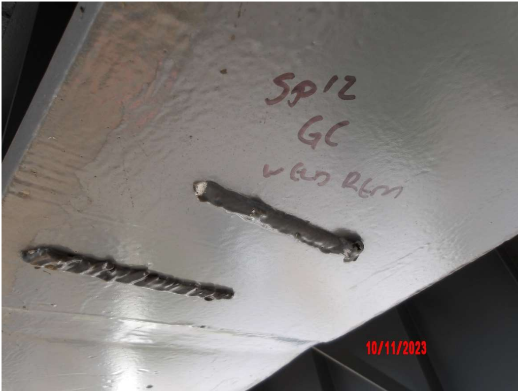
Photo 40- Girder C, Span 12, Typical Weld Remnants on Bottom Flange
