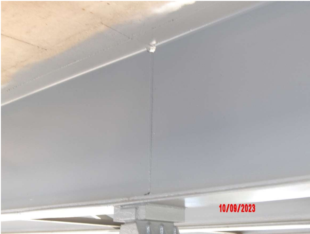
Photo 32- Girders at Pier 1, Typical Web Weld with Holes
