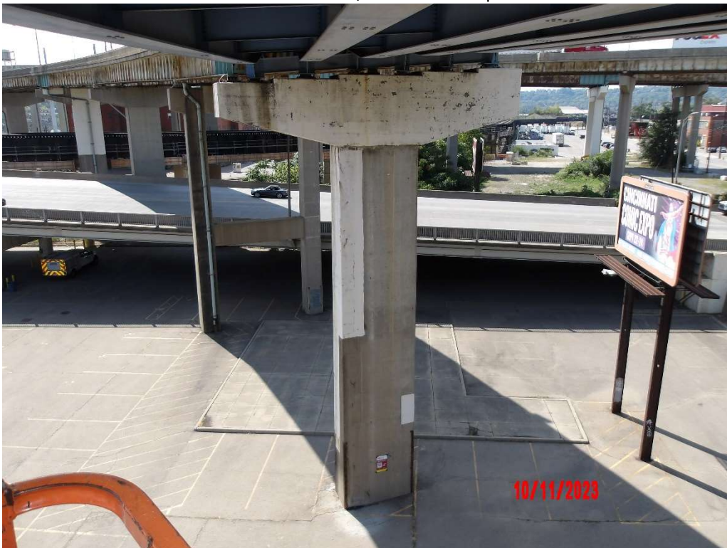
Photo 85- Pier 20D Front Face, Note FRP Wrap Delaminations
