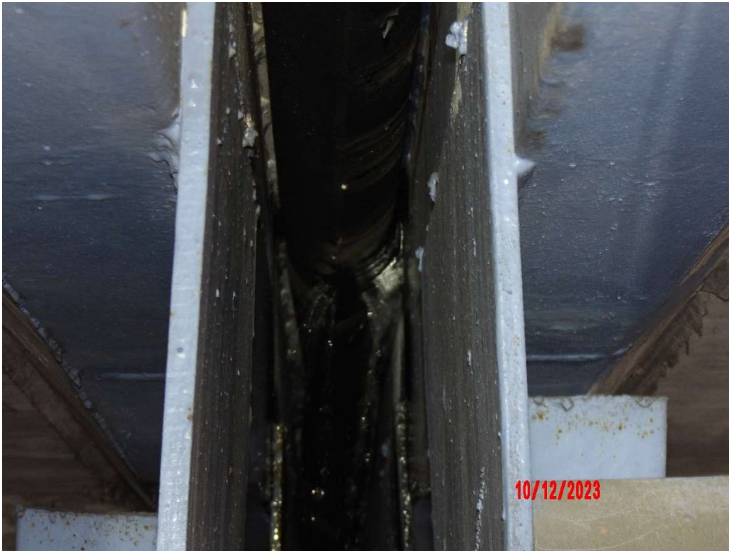
Photo 18- Pier 25C, Joint Tear, Free Flow Water
