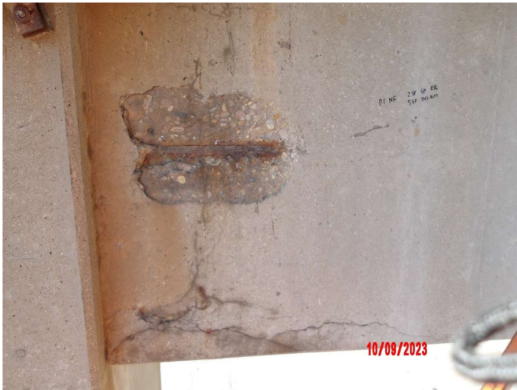
Photo 86- Pier 1, North Face Cap, Spall 2SF, Delaminations 5SF
