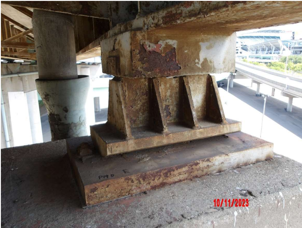
Photo 55- Pier 19D, Bearing E, Minor Corrosion
