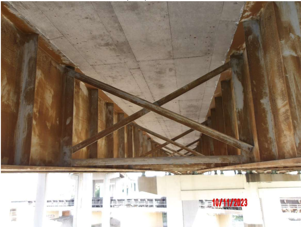
Photo 45- Span 15, Typical Condition, Paint Failure
