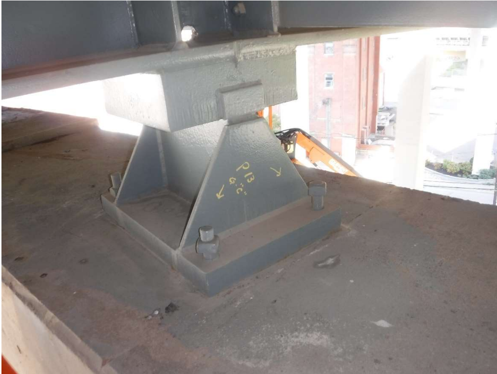
Photo 58- Pier 13, Bearing C, Loose Anchor Bolts
