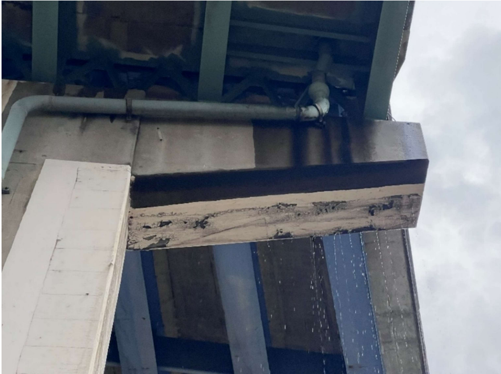
Photo 26- Drainage, Leaking on Substructure, Pier 25
