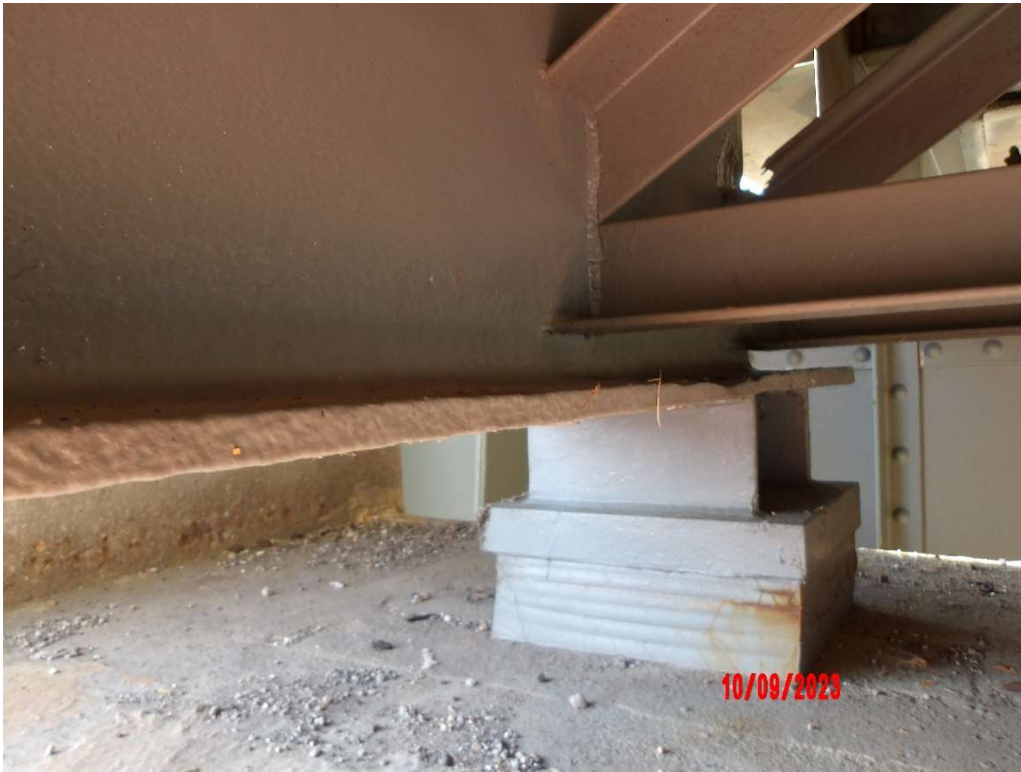
Photo 30- Girder G, Pier 0, Bottom Flange and Web, Up to 3/8" Section Loss, 9' L
