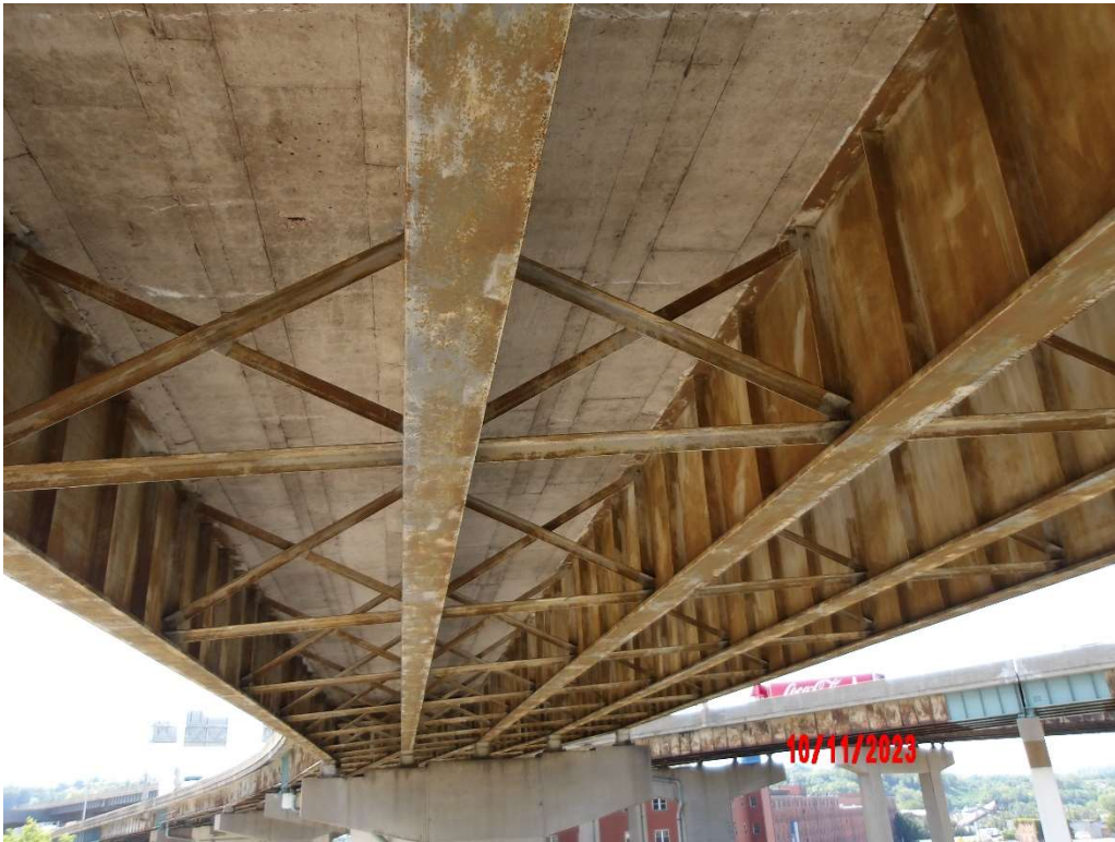
Photo 46- Span 19, Typical Condition, Paint Failure
