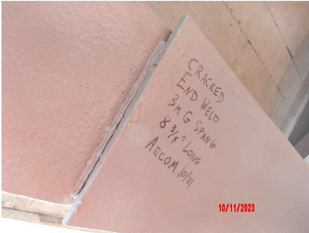
Photo 38- Girder G, Span 6, Completely Cracked End Weld on Bottom Flange
