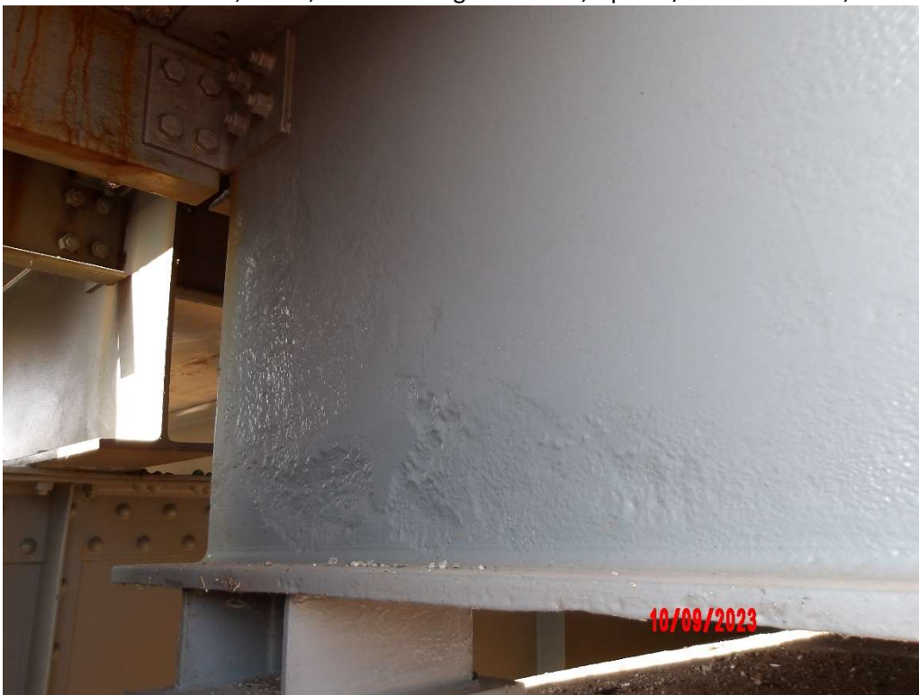
Photo 31- Girder G, Pier 0, Bottom Flange and Web, Up to 3/8" Section Loss, 9' L
