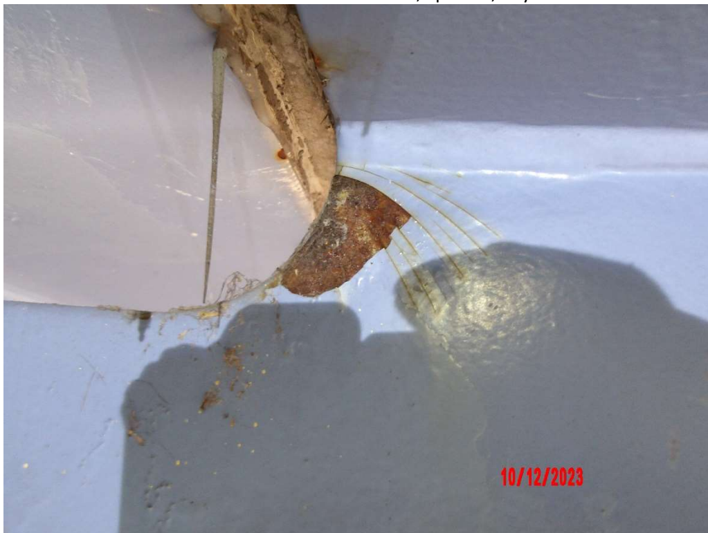
Photo 70- Cross Frame, Span 24, Bay 3, Coping Detail with Paint Cracking
