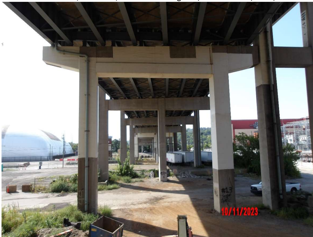
Photo 82- Pier 12 FF, FRP Wrap Delaminations
