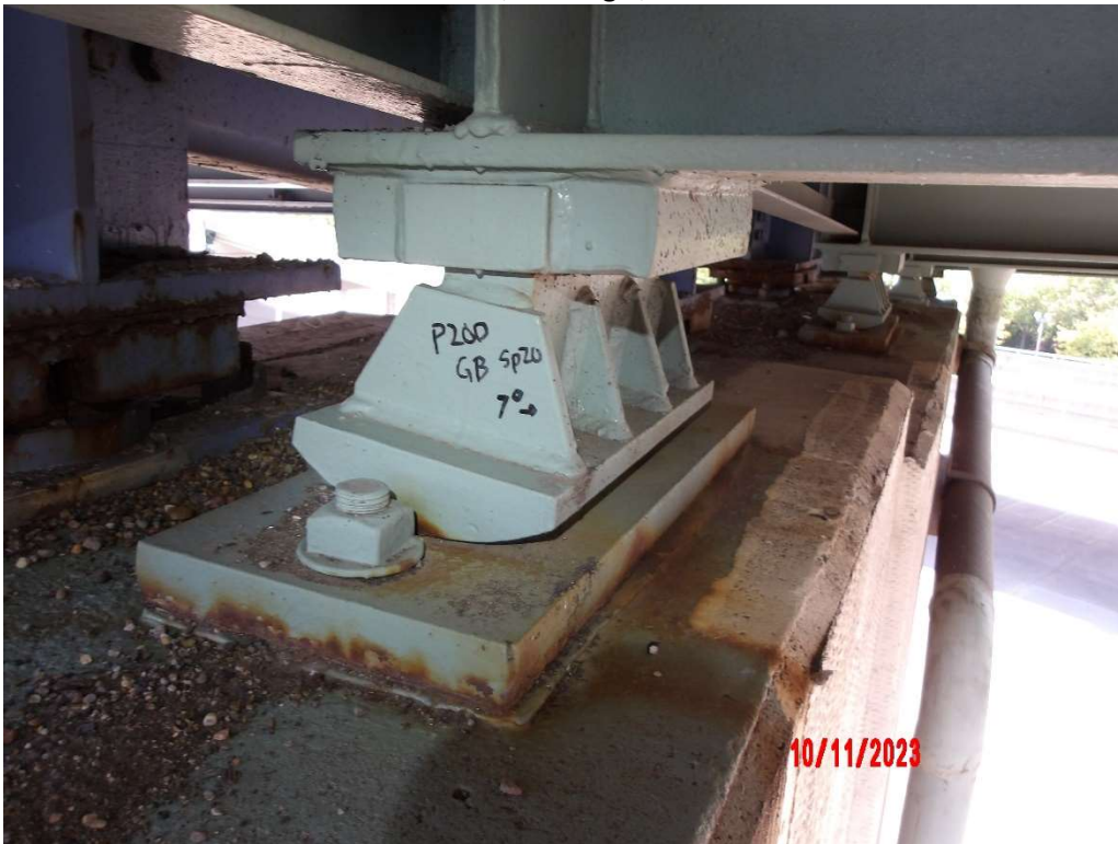
Photo 56- Pier 20D, Bearing B, Span 20, 7 degree in contraction.
