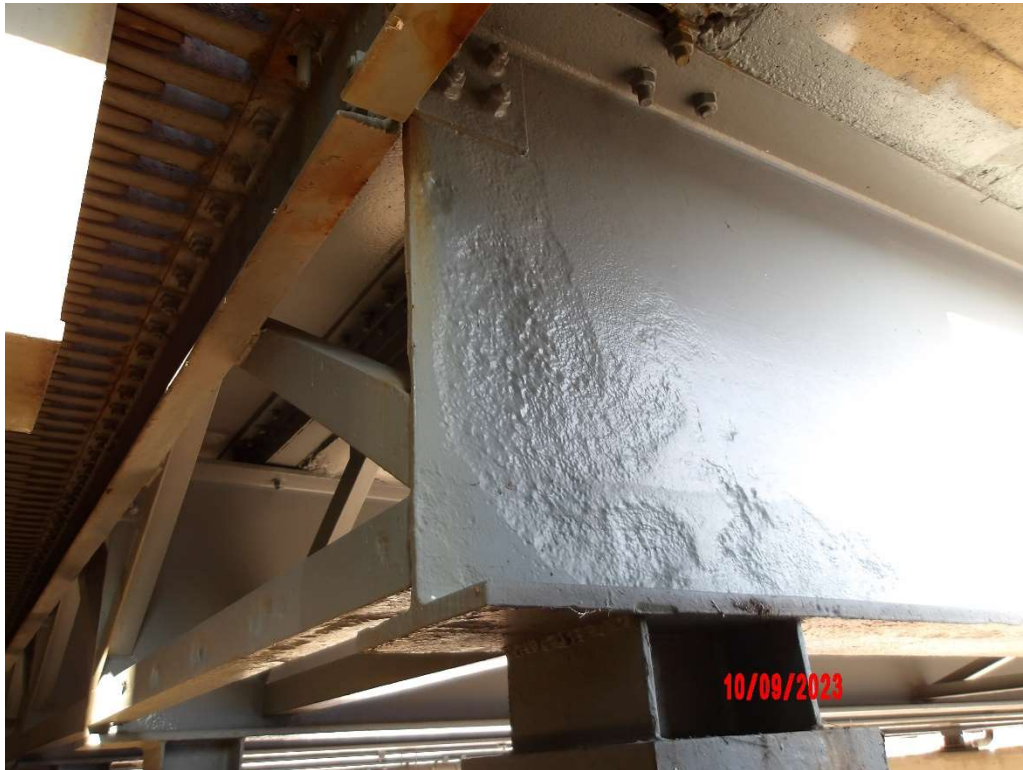
Photo 27- Girder A, Pier 0, Bottom Flange and Web, Up to 3/8" Section Loss, 9' L
