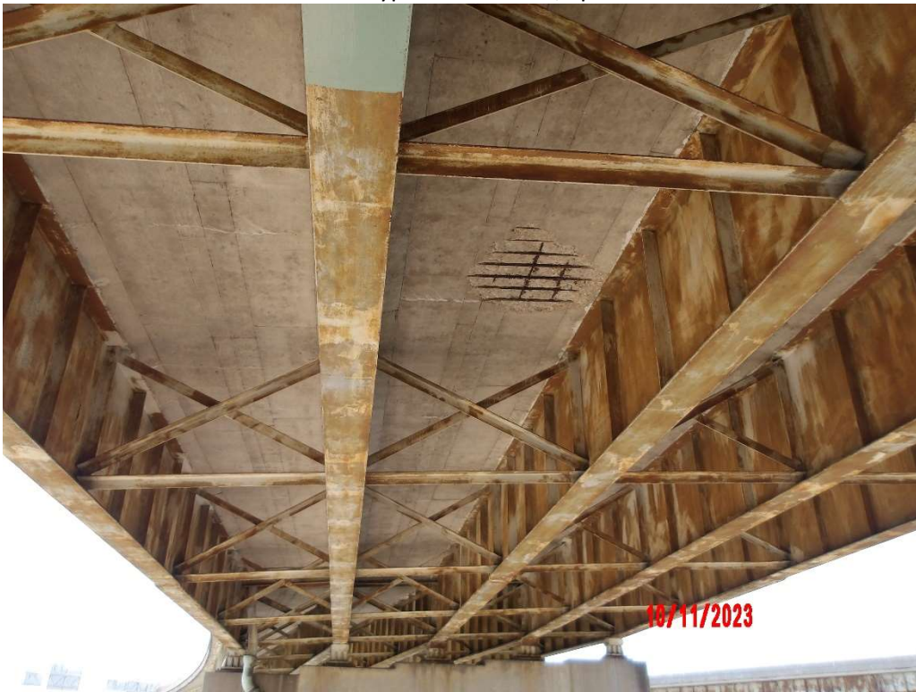
Photo 8- Typical Underside, Span 20, Spalling with Exposed Rebar
