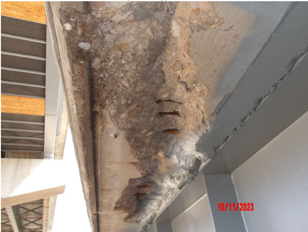
Photo 6- Girder A, Span 14, 8'x7'x6" Spall with Exposed Rebar
