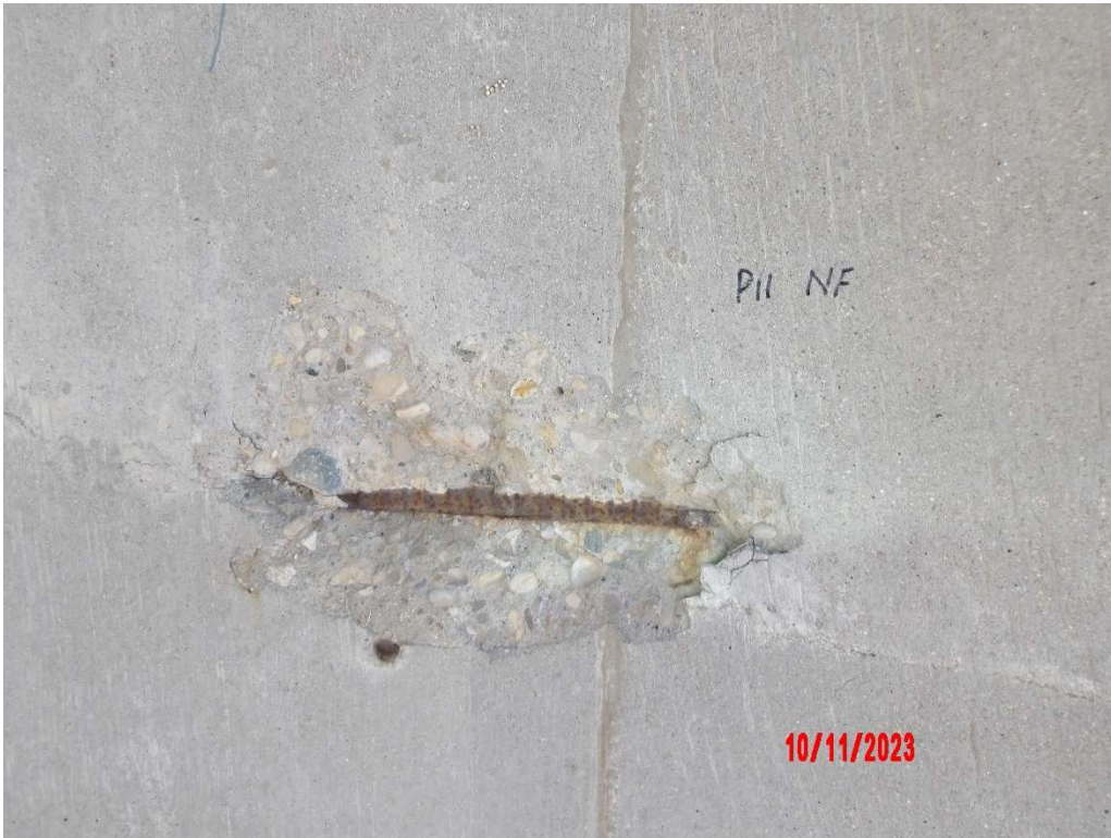
Photo 93- Pier 11, Northface of Cap, 2 SF Spall with Exposed Rebar
