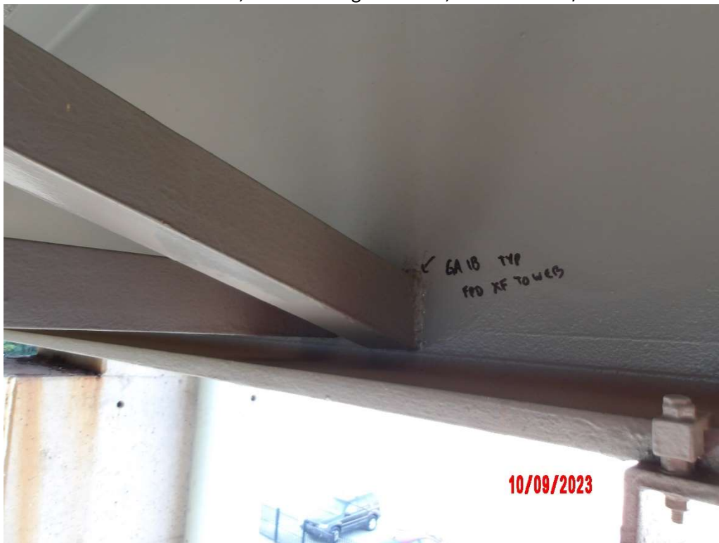
Photo 35- Girder A, Span 5, Inboard, Typical Cross Frame Weld to Web
