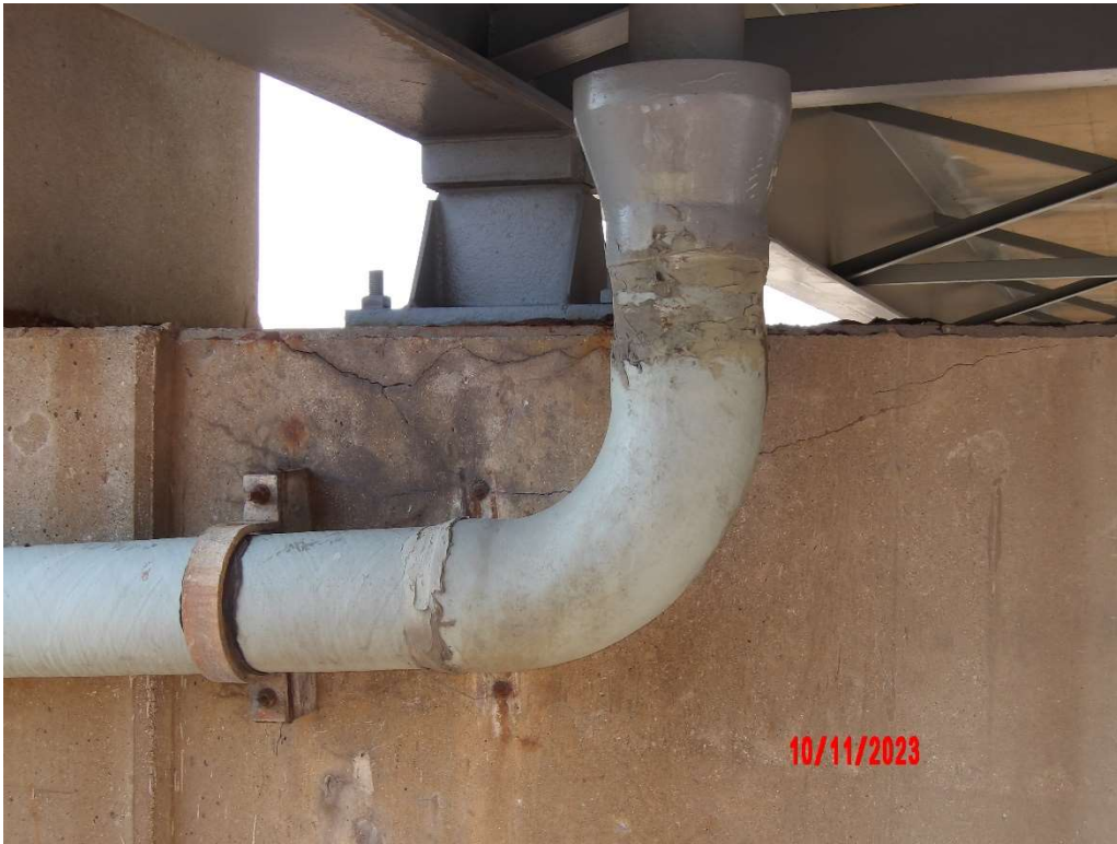
Photo 91- Pier 6, Cap North Face, 6 SF Cracking \sim 1/32 " Wide
