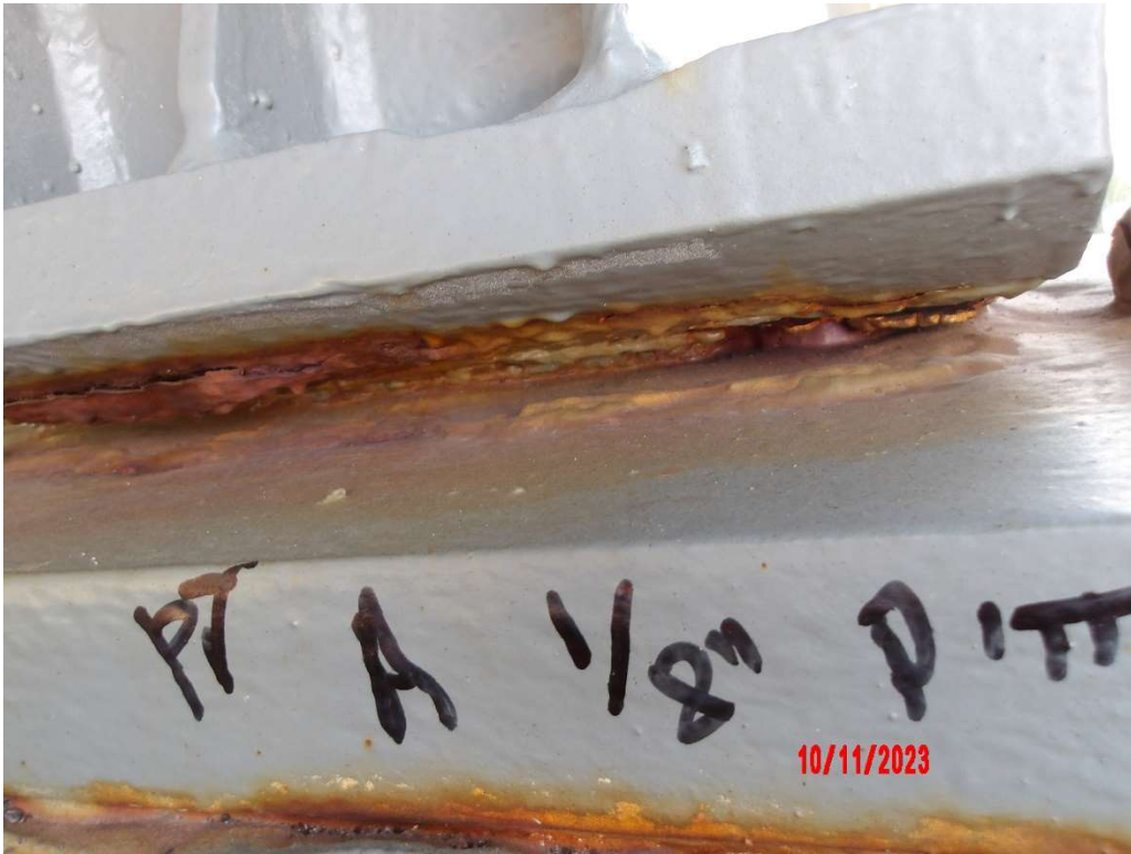
Photo 51- Pier 7 Bearing A, 1/8" Pitting
