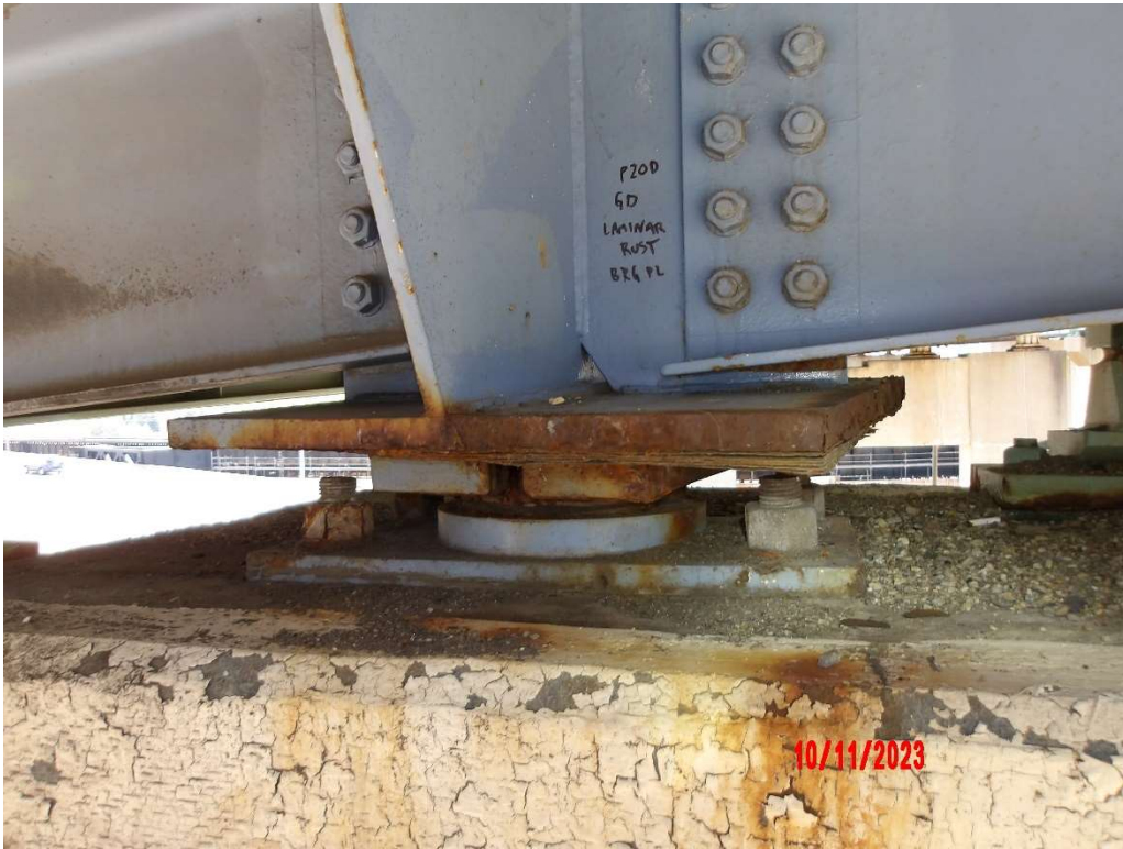
Photo 60- Pier 20D, Bearing D, Typical Laminar Rust, 1/8" SL Bearing Plate
