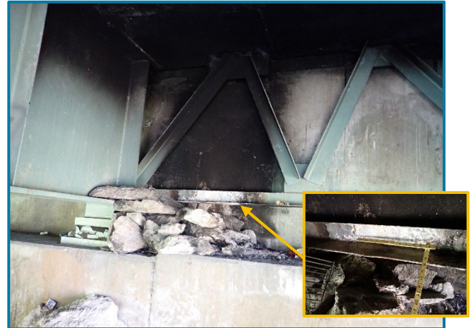
Photo 18 – Fire damage to the end crossframe between Girders C and D at Abutment A (looking northwest).
