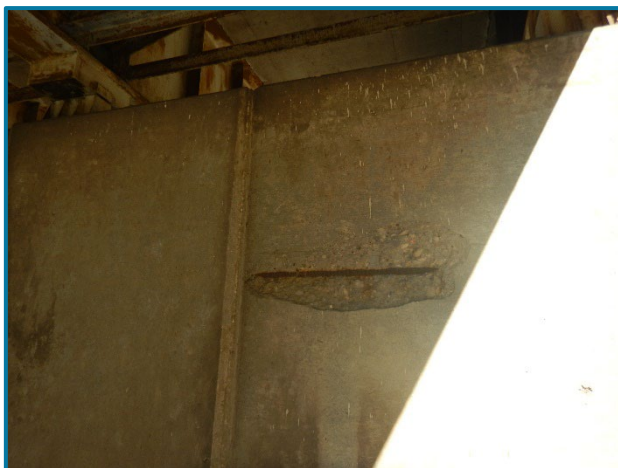
Photo 25 – 2' wide by 1' high by 2" deep spall with exposed reinforcement on the south face of the Pier 21A cap between Girders D and E (looking north).
