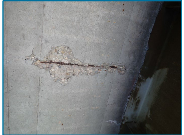
Photo 3 - 24" wide by 12" long by 1" deep spall with exposed reinforcement in the deck underside between Girders D and E in Span 24A (looking south).
