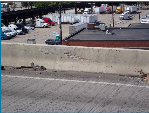
Photo 8 – Shallow spall on the interior face of the west railing in Span 22A at midspan (looking west).
