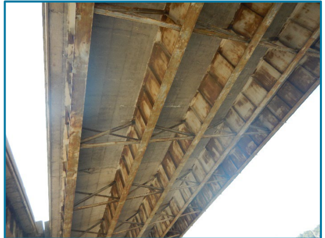
Photo 16 – Typical steel protective coating condition of all steel members in Span 21A (looking southwest).
