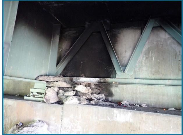
Photo 27 – Fire damage with discoloration and cracking on the Abutment A backwall between Girders C and D (looking northwest).
