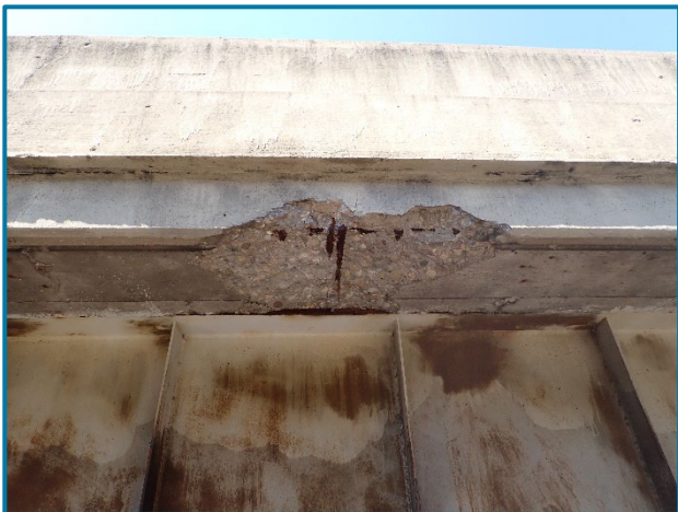
Photo 4 - 36" long by 24" wide by 4" deep spall with exposed reinforcement in the east overhang in Span 22A (looking west).
