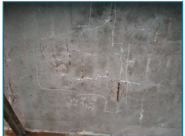
Photo 5 - 8' long by 8' wide by 1" deep spall with exposed reinforcement and surrounding delaminations in the deck underside between Girders B and C in Span 23A (looking south).
