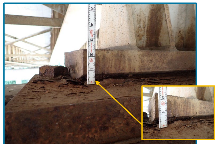
Photo 12 – 1/4" thick pack rust between the masonry plate and rocker bearing of Girder E at Pier 20A (looking southwest).
