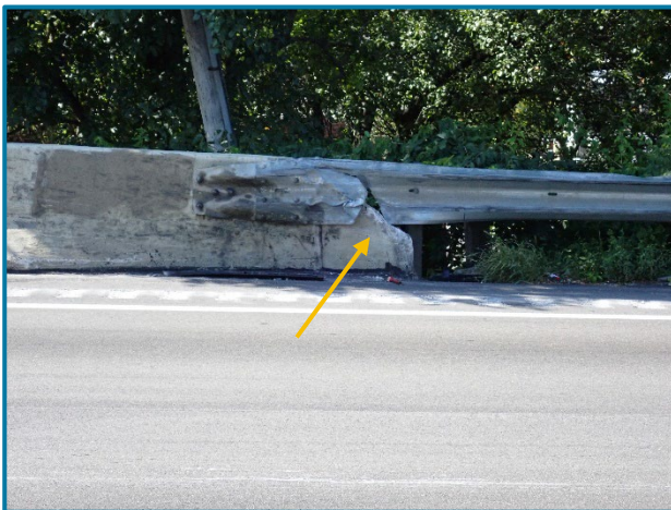
Photo 29 – Impact damage to the approach guardrail at the transition to the concrete railing on the west side of the north approach (looking west). Note the spall at the end of the concrete railing.
