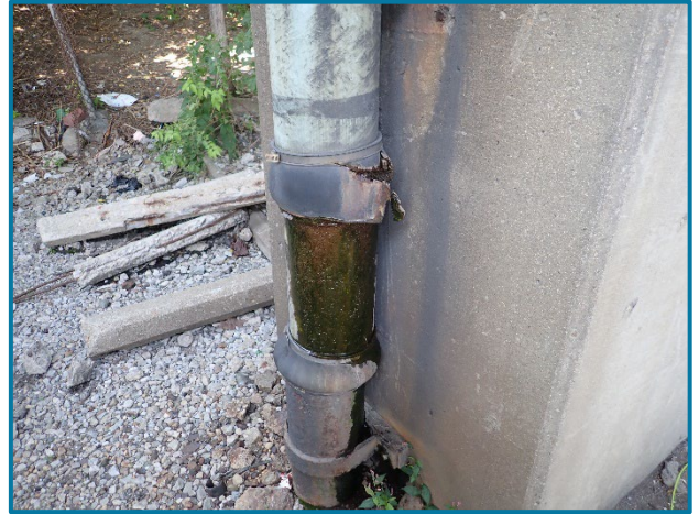
Photo 10 – Bulging and cracked drainage coupling gasket at the base of Column 1 on the south face of Pier 23A (looking northwest).
