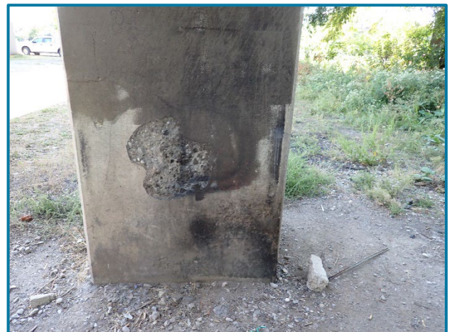
Photo 22 – 20" diameter by 1" deep spall on the north face of Column 2 at Pier 23A (looking south near the base).
