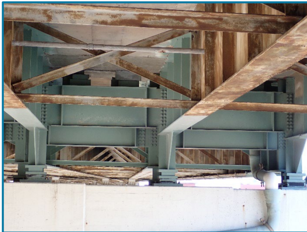
Photo 15 – Typical steel protective coating condition of the girder ends at Pier 19A (looking southeast).
