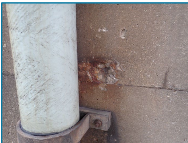
Photo 21 – 6" diameter spall near the drainage support bracket on the south face of Column 1 at Pier 23A (looking north about 15' above the ground).
