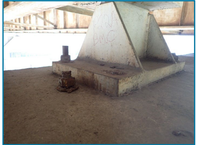
Photo 14 – One broken anchor bolt at the northeast corner of the Girder C bearing at Pier 22A (looking southwest).
