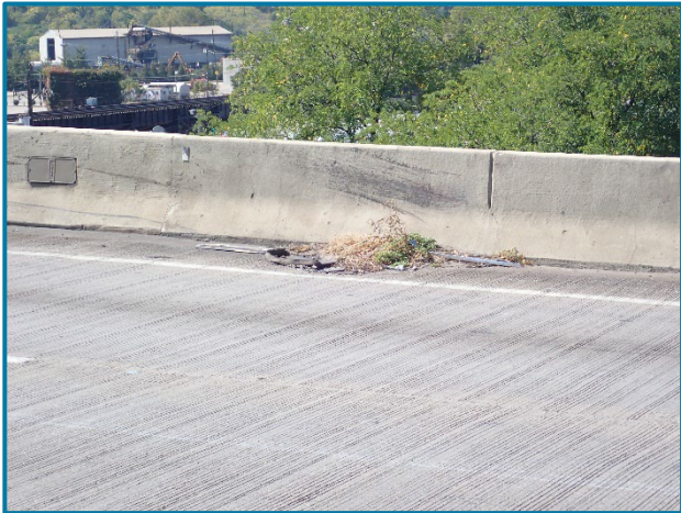
Photo 9 – Clogged scupper in the west shoulder on the top of deck at Pier 23A (looking southwest).
