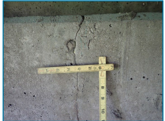
Photo 23 – Isolated vertical hairline crack in the abutment seat below Girder B in Span 25A (looking north at the south face of Abutment A).
