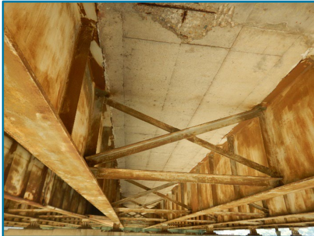
Photo 17 – Typical crossframe with minor surface corrosion and paint failure (looking south in Span 21A between Girders D and E).
