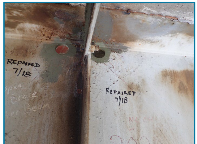
Photo 19 – Typical crack arrest hole repairs in east face web of Girder C at the midspan crossframe connection (looking west in Span 23A).
