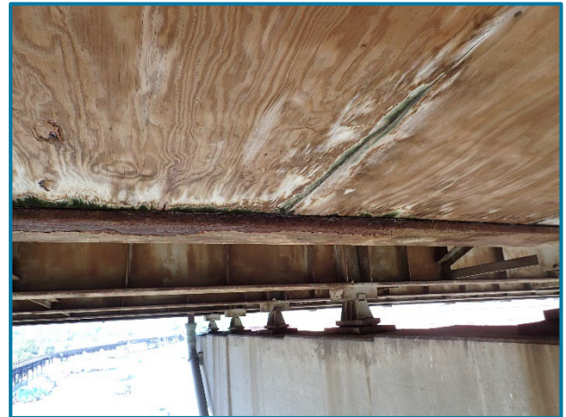
Photo 11 – Laminate corrosion with up to 1/8" section loss in the bottom flange of Girder E in Span 20A near Pier 20A (looking east).
