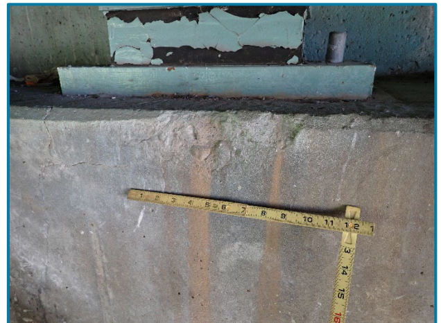
Photo 24 – Shallow edge spall on the Abutment A bearing seat at Girder D (looking north).
