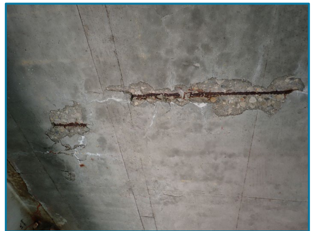
Photo 1 – Isolated delamination/spall with exposed reinforcement and adjacent typical hairline transverse cracks in the deck underside (looking up and south between Girders B and C in Span 23A).
