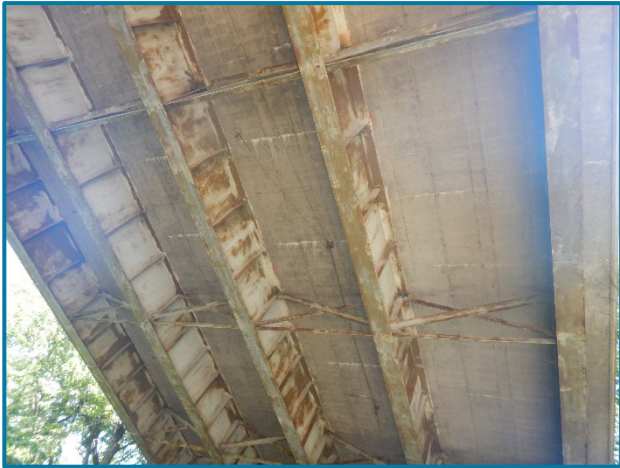
Photo 2 - Typical transverse cracks throughout the deck underside in the interior bays in Span 24A (looking northwest).
