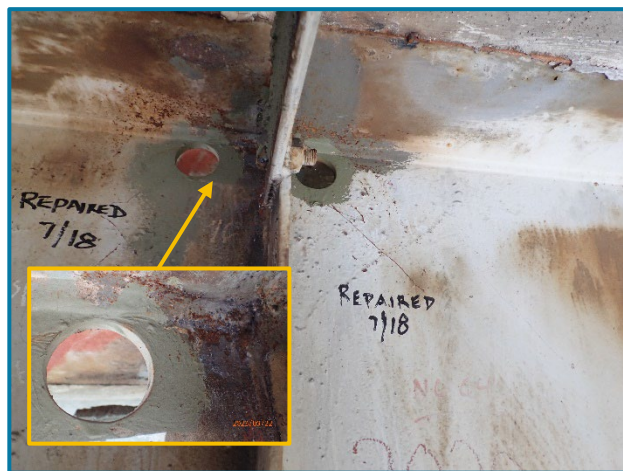
Photo 13 – Typical crack arrest hole in the web of Girder C near top flange (looking west in Span 23A at midspan).
