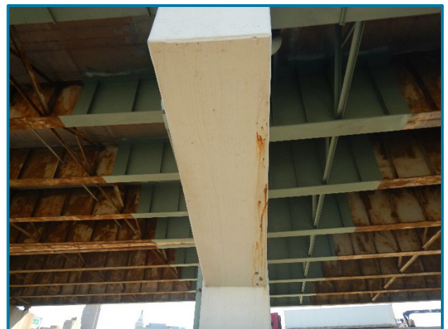
Photo 26 – Area of delamination, cracking, and rust staining on the underside of the Pier 19A cap (looking east at the west end of the cap).
