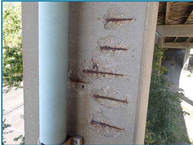
Photo 20 – Spalls with exposed reinforcement on the south face of Column 1 at Pier 22A (looking north).
