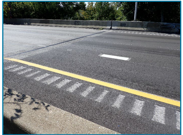
Photo 28 – New asphalt wearing surface overlay on the north approach slab (looking southwest).
