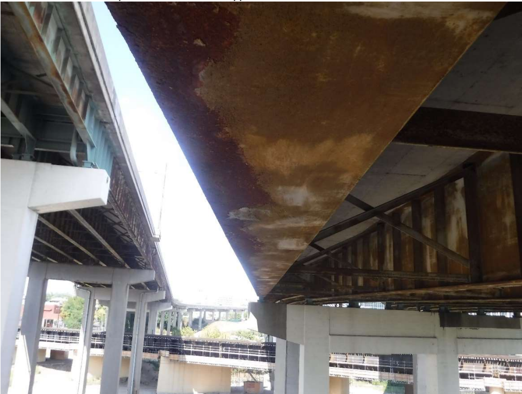
Photo 18- Span 15, Girder A, Typical Paint Failure and Active Corrosion
