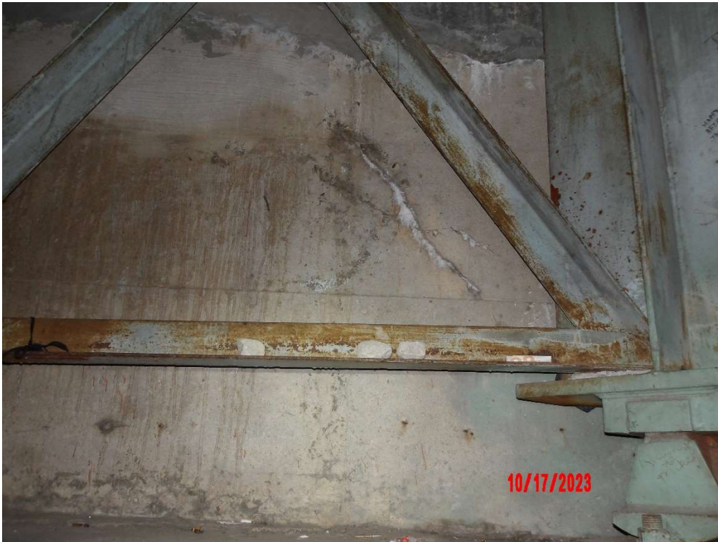
Photo 47- Abutment C, Bay 4, Crack in Backwall
