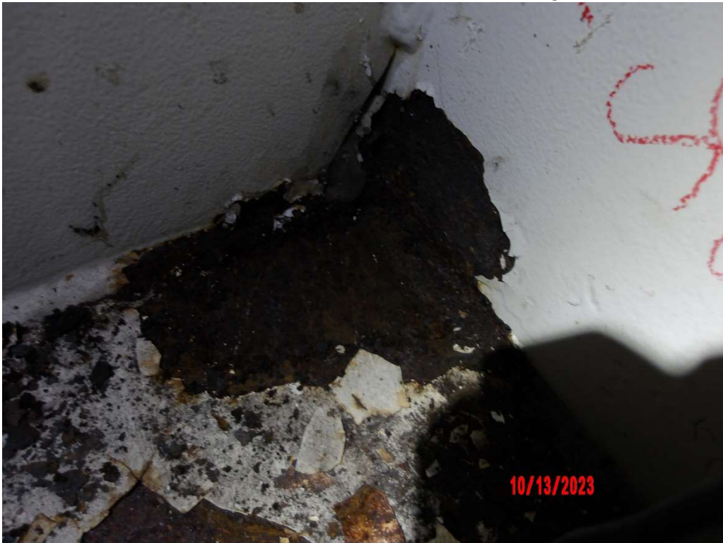
Photo 62- Pier 26J, South Web, Stiffener 17, Moderate Corrosion,
