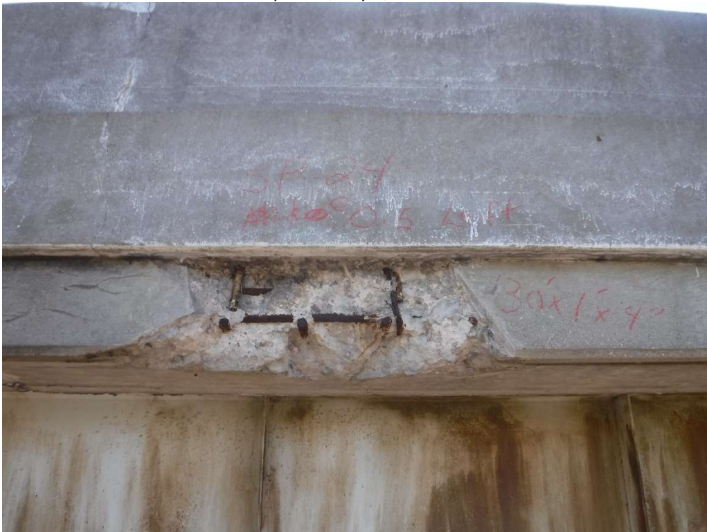
Photo 9- Span 24, Overhang, Spall with Exposed Rebar
