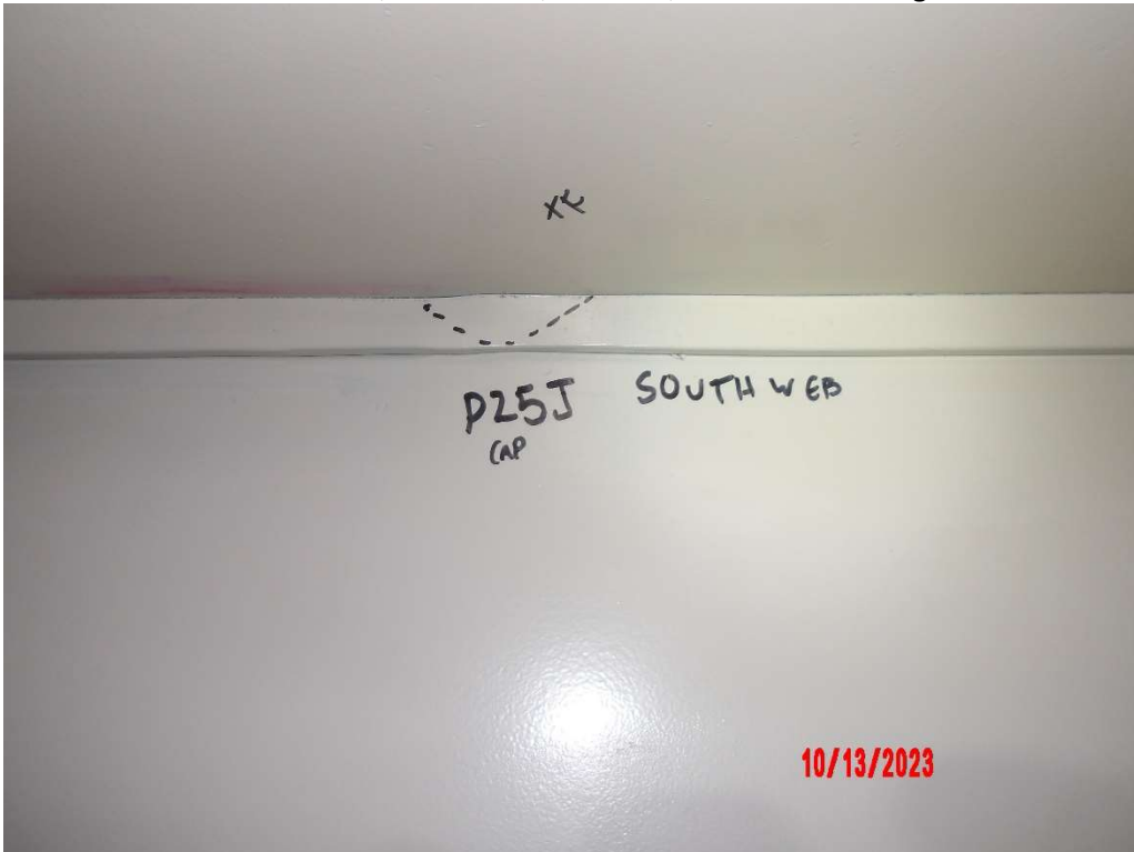
Photo 53- Pier 25J, South Face, Deformed Backing Plate
