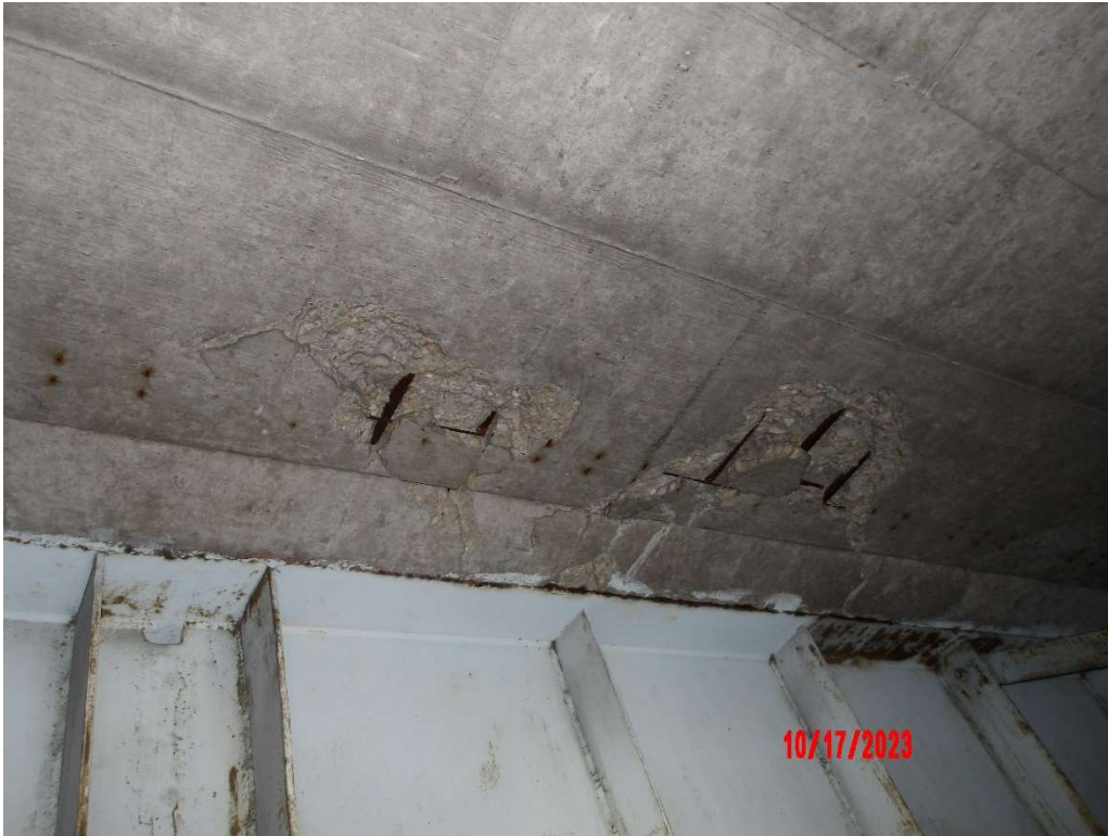
Photo 10- Span 29, 9SF Spall with Exposed Rebar
