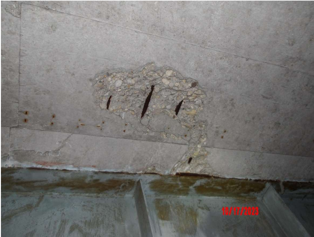
Photo 12- Span 29, Bay 1, 5SF Spall with Exposed Rebar
