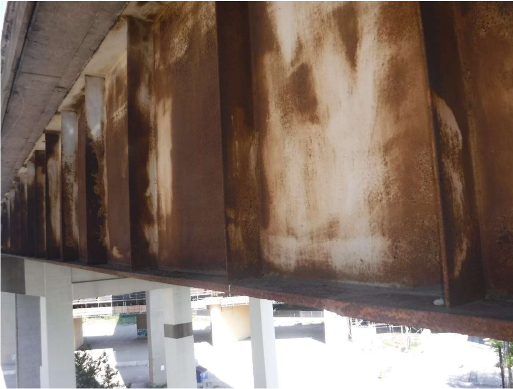
Photo 17- Span 15, Girder A, Typical Paint Failure and Active Corrosion
