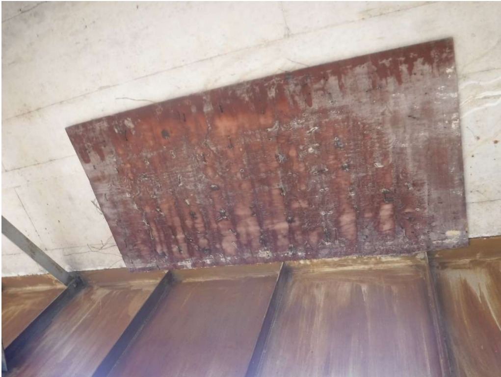
Photo 8- Span 24, Bay 1, Form Remnants
