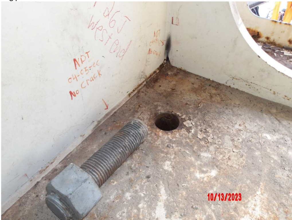
Photo 25- Pier 26J, West End, Bearing Anchor Bolt Removed
