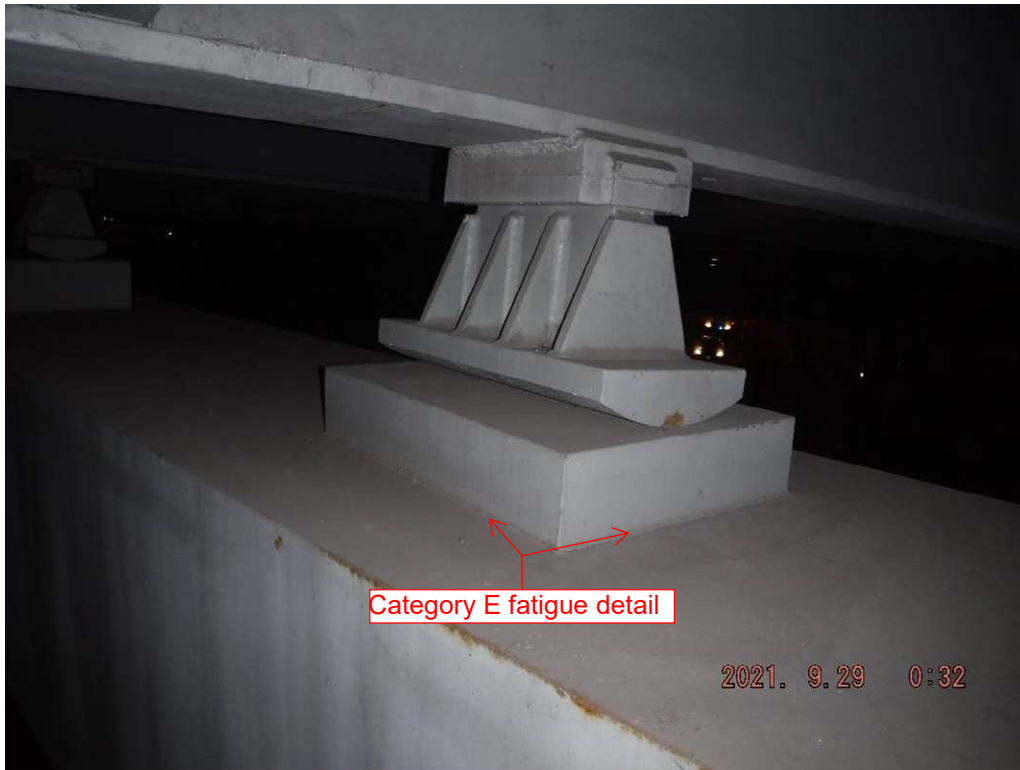
Photo 56 - Category E fatigue detail - Steel bearing pedestal welded to top flange
