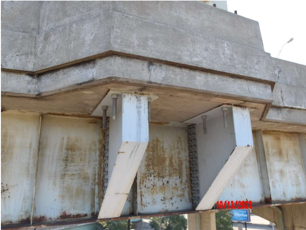
Photo 6- Span 23J, Sign Bumpout Detail
