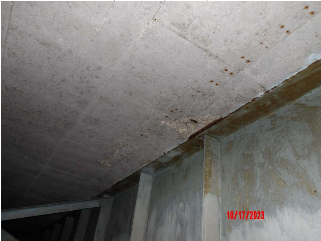
Photo 11- Span 29, Bay 1, 2SF Spall with Exposed Rebar
