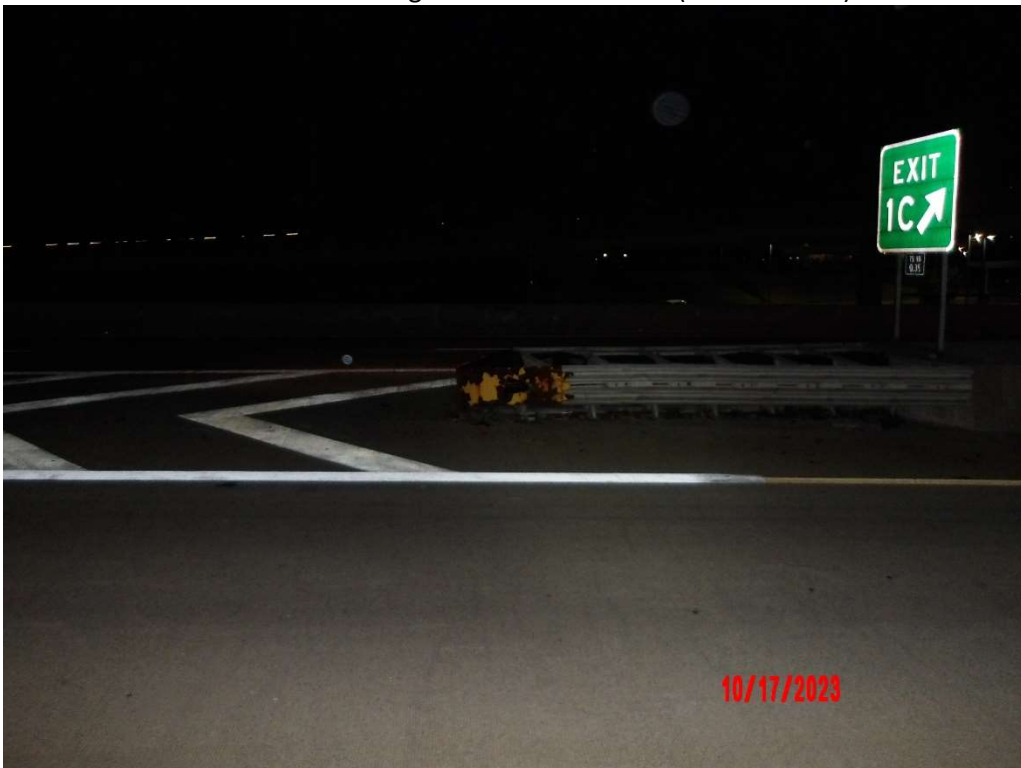
Photo 15- Deck, Smashed Attenuator on Guardrail near Exit 1C
