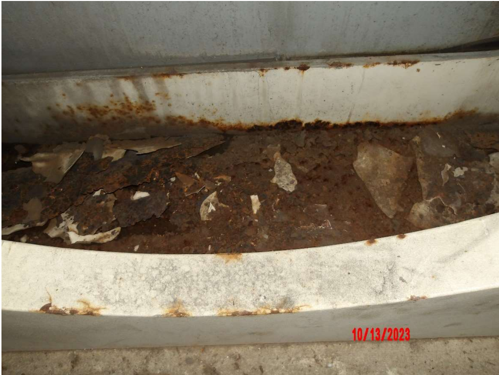
Photo 61- Pier 26J, East End, Moderate Corrosion to Bottom Flange with Paint Failure
