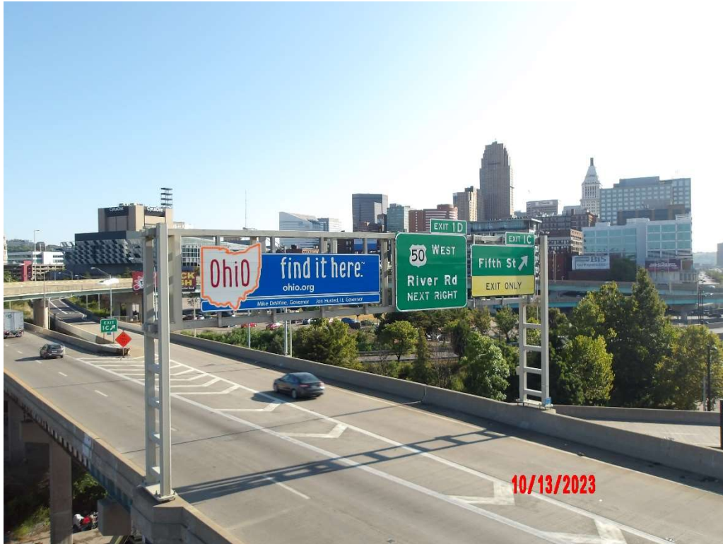
Photo 13- Typical Wearing Surface Conditions
