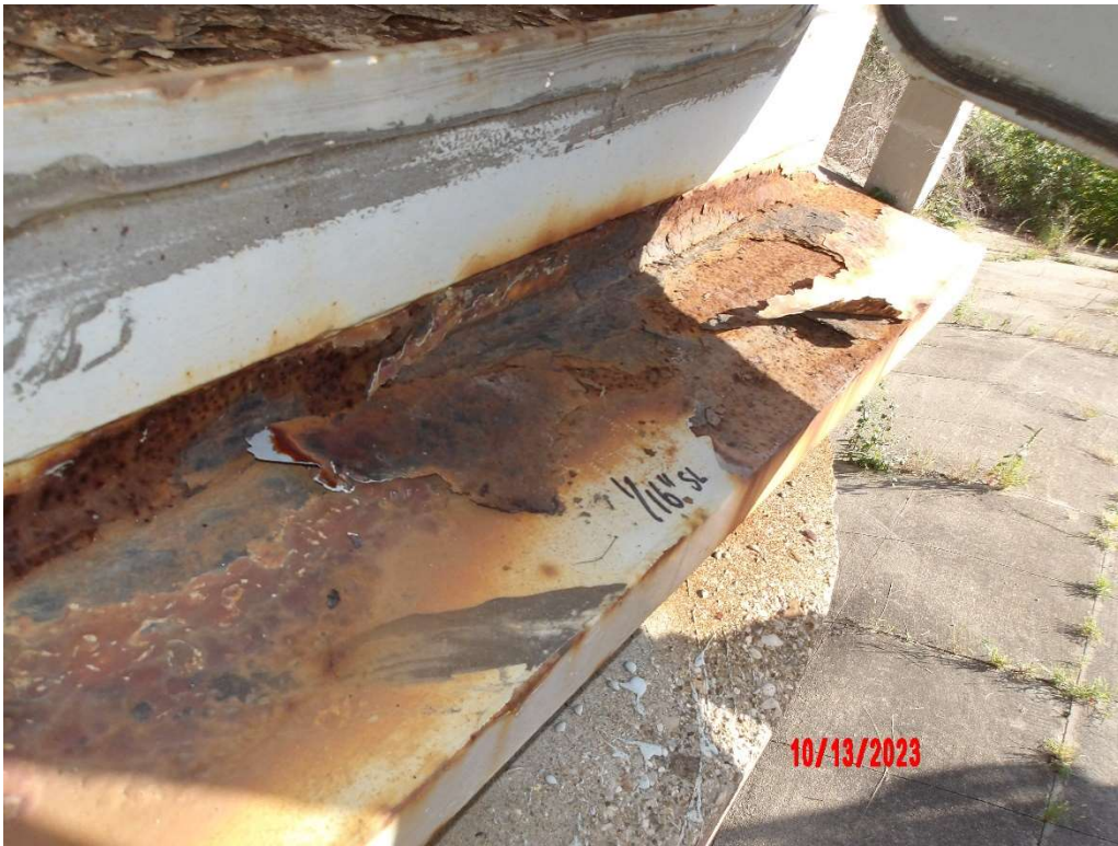
Photo 60- Pier 26J, West End, Up to 1/16" Section Loss Bottom Flange
