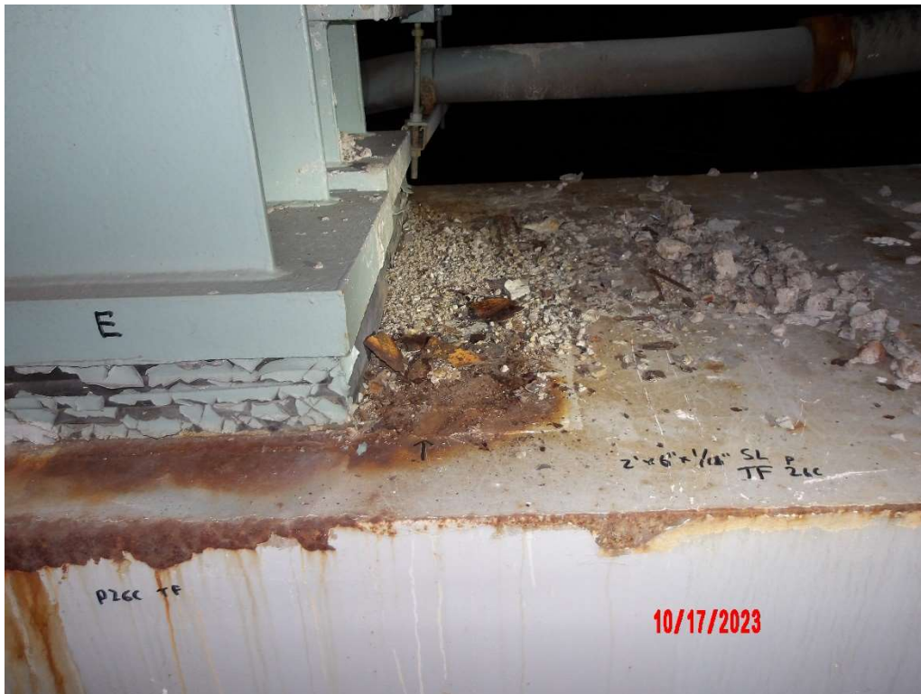
Photo 57- Pier 26C, Top Flange, 2' x 6" x 1/16" SL
