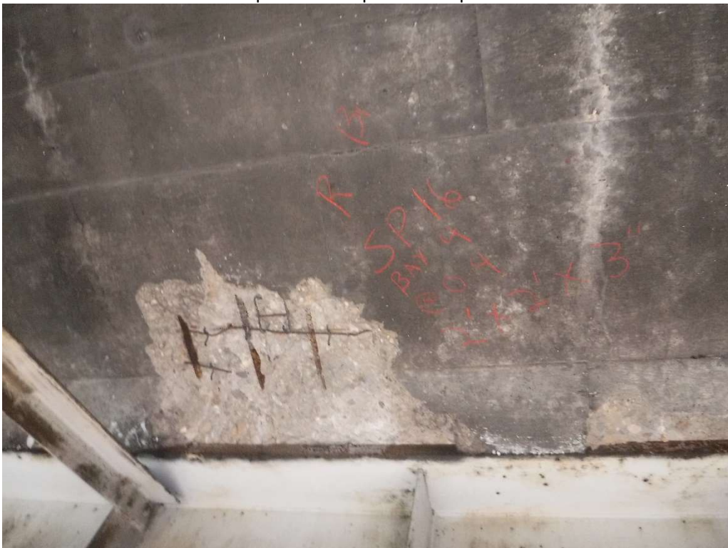
Photo 5- Span 16, Bay 4, 4SF Spall with Exposed Rebar
