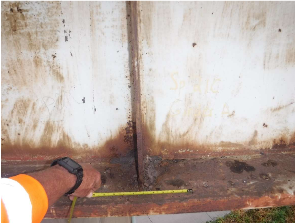
Photo 21- Girder A, Span 21C, Bottom Flange Section Loss, 1'x6"x1/8"
