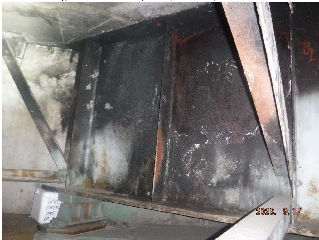
Photo 24- Fire Damage under Structure, Bay 3, Span 29
