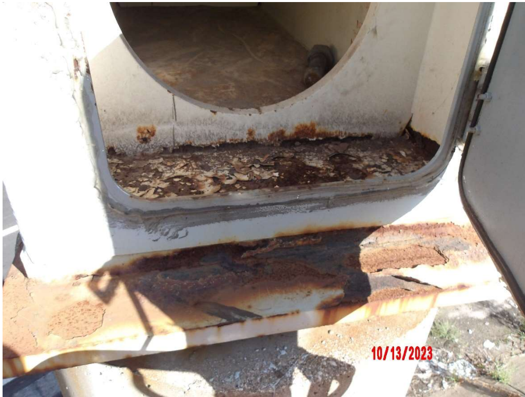
Photo 65- Pier 26J, West End, Moderate Corrosion to Bottom Flange with Paint Failure
