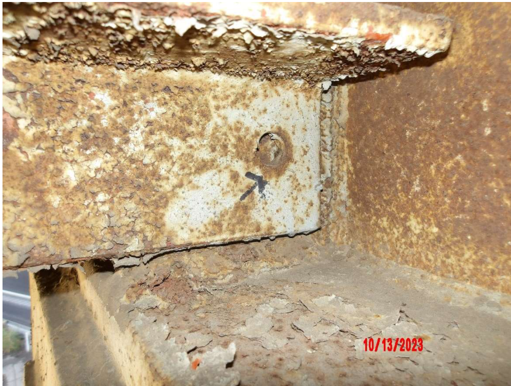
Photo 39- Span 26, Cross Frame, Missing Bolt Typical
