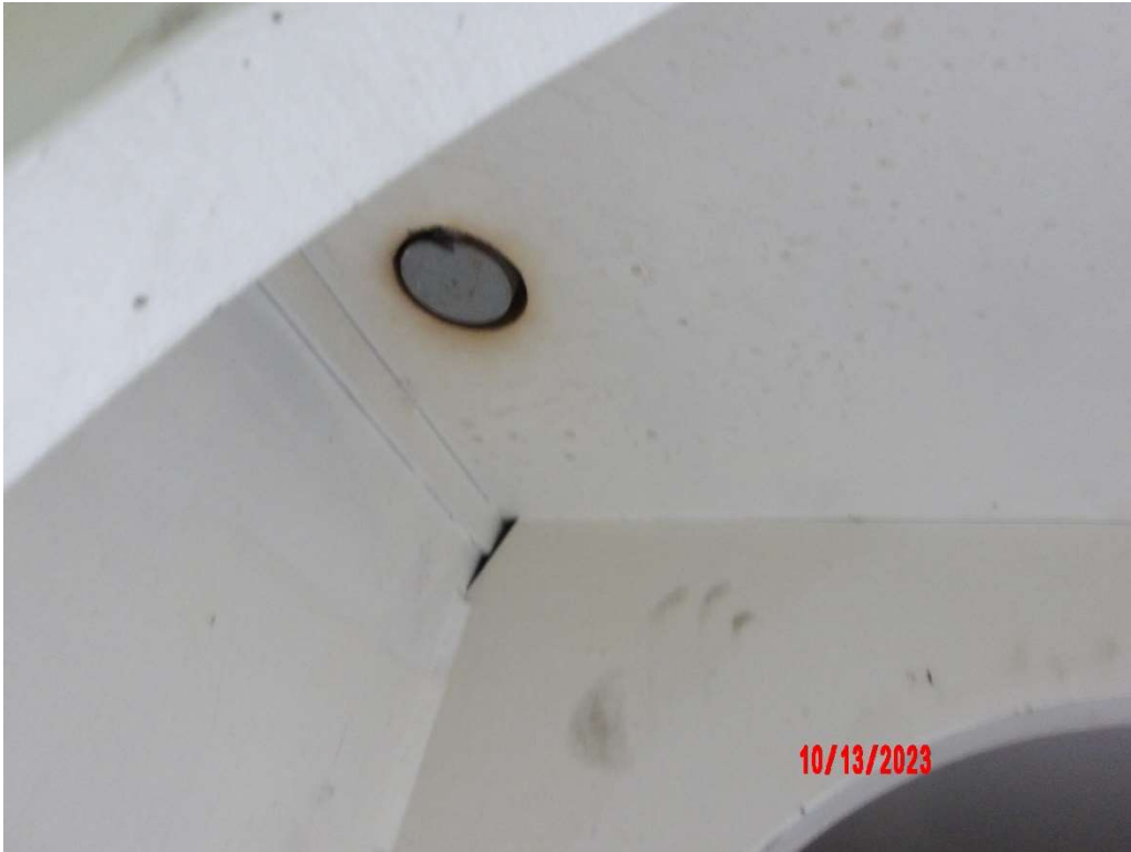
Photo 63- Pier 26J, Stiffener 12, Drill Holes in Top Flange
