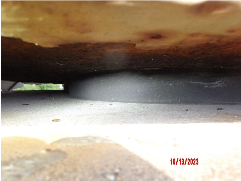
Photo 26- Pier 26J, West End, Bearing Slight Bulge at Opposite Location of Missing Bolt
