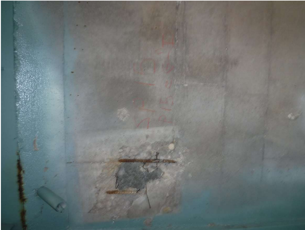
Photo 4- Span 15 2SF Spall with Exposed Rebar
