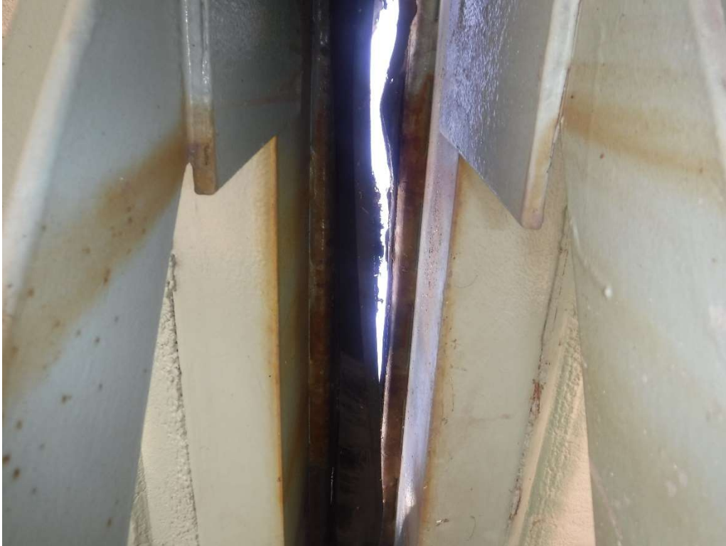
Photo 14- Joint Failure, Pier 23 near Girder E
