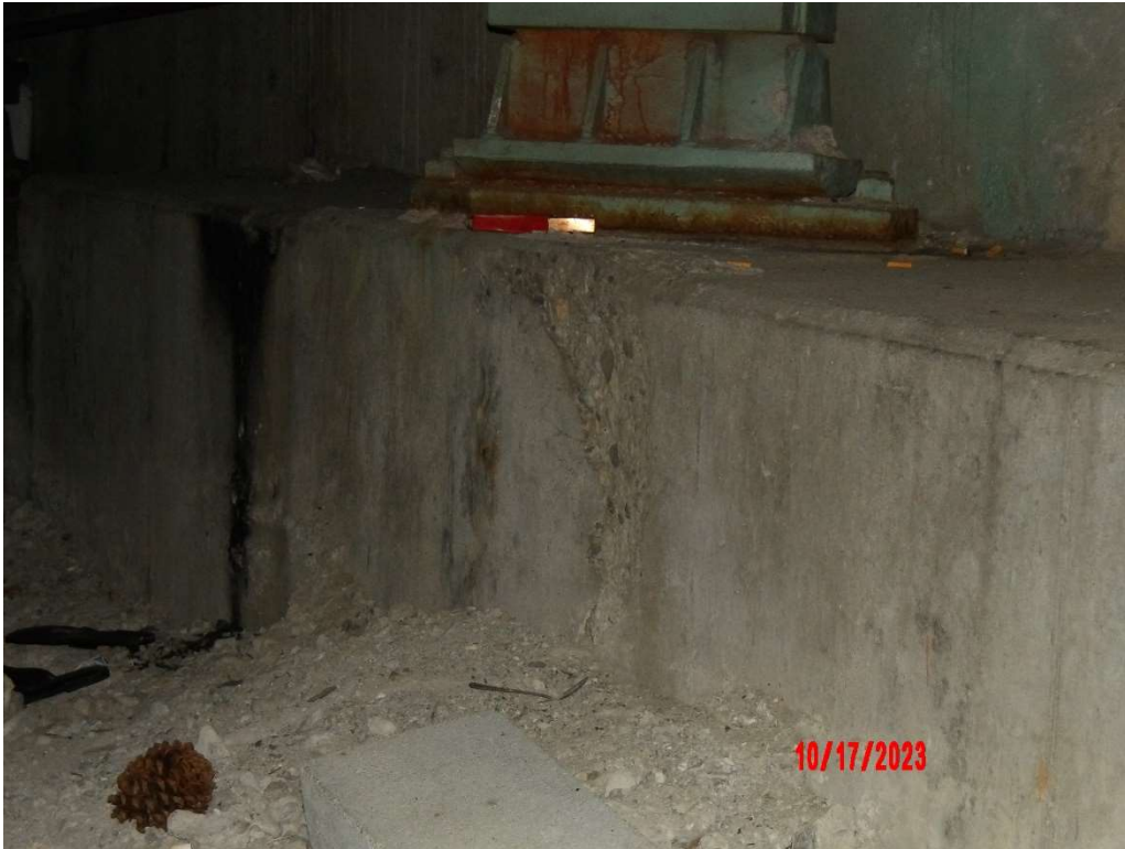
Photo 48- Abutment C, Bearing D, Spall in Abutment
