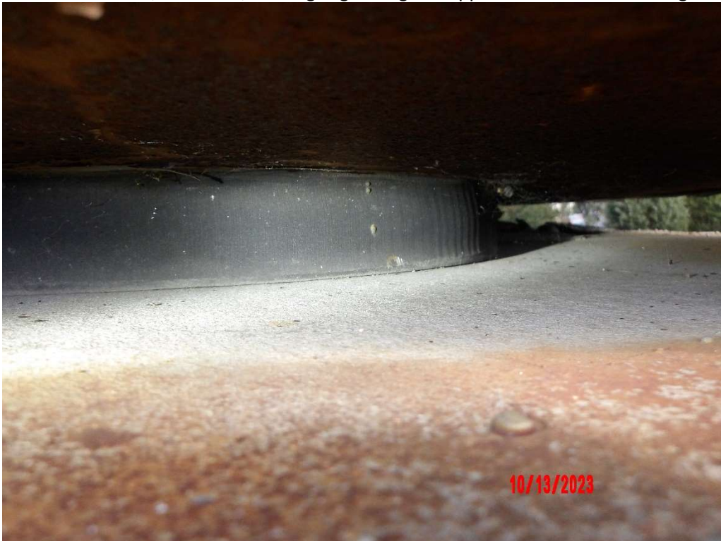
Photo 27- Pier 26J, West End, Bearing Slight Gap under Bearing at Location of Missing Bolt
