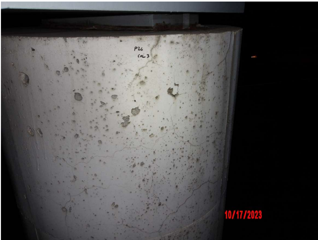
Photo 46- Pier 26J, Column 3, Heavy Map Cracking
