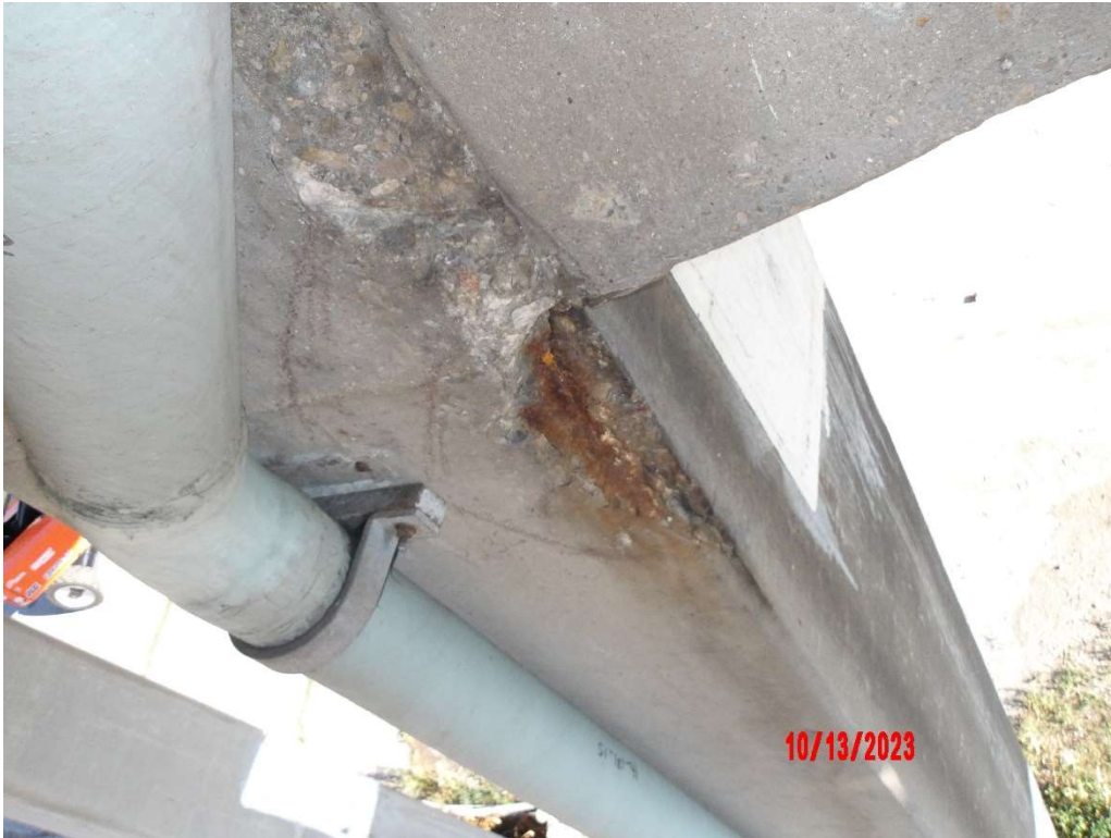
Photo 45- Pier 23C, Column 3, Spall with Exposed Rebar 3SF
