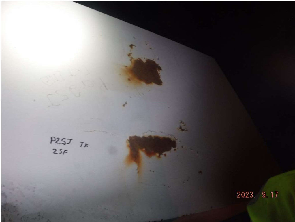
Photo 51- Pier 25J, Top Flange, 2 SF Active Corrosion
