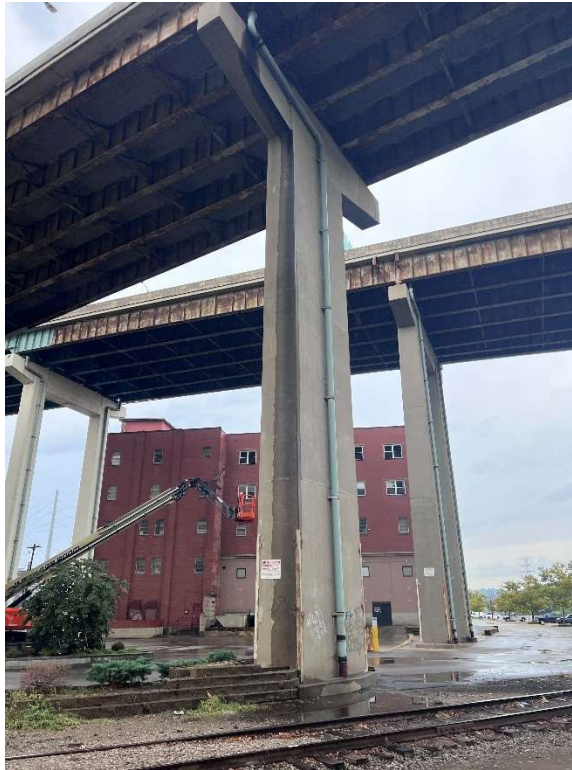
Photo 16- Drainage, Leaking on Substructure, Pier 16C
