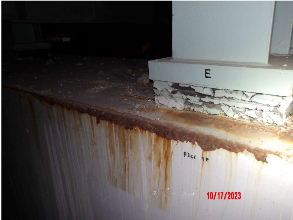
Photo 58- Pier 26C, Top Flange, Active Corrosion
