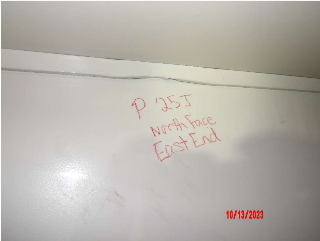
Photo 52- Pier 25J, North Face, East End, Deformed Backing Plate
