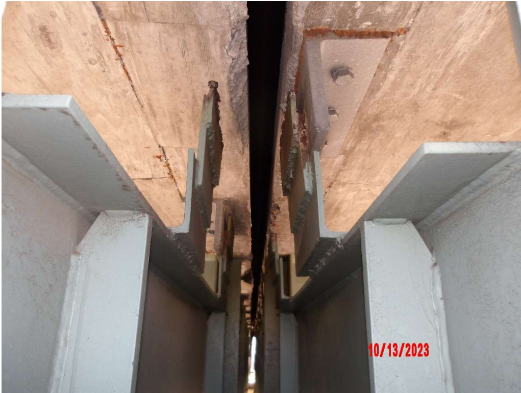
Photo 37- Cross Frames, Pier 23J, Welded Retrofit for Joint Replacement Remnants
