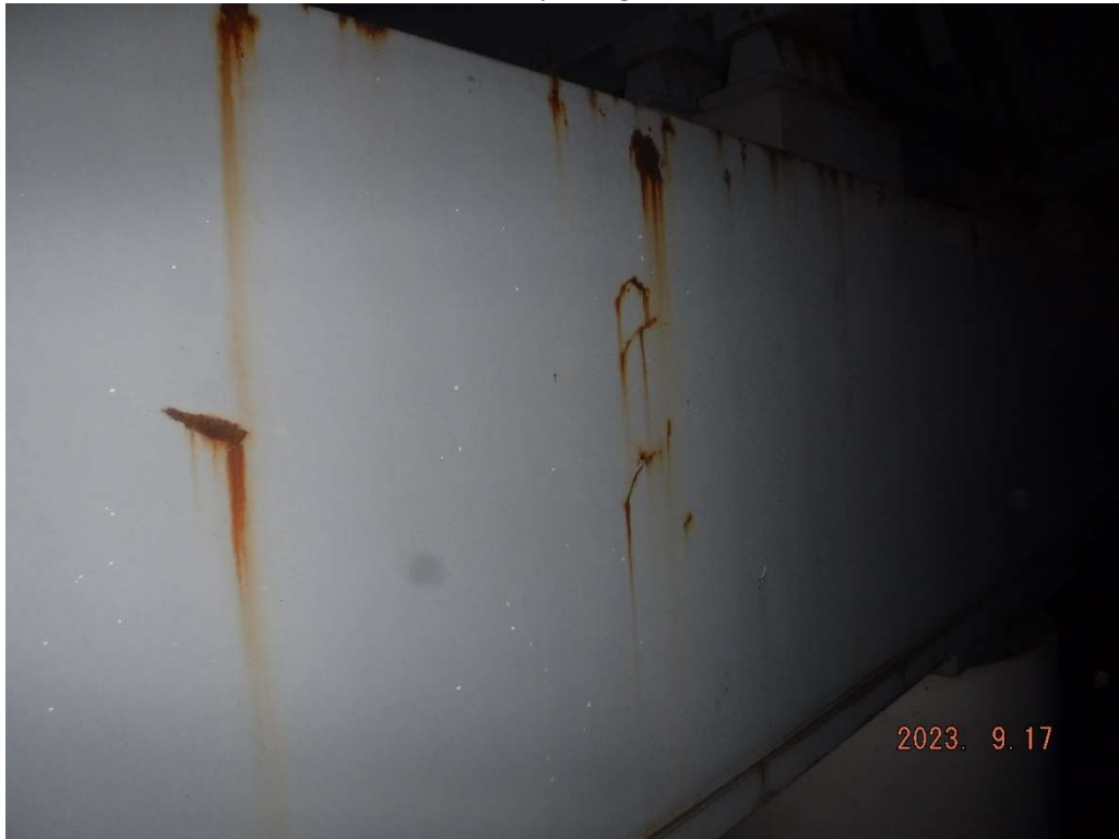
Photo 59- Pier 26C-Pier 26J, South Face, Scrapes and Active Corrosion
