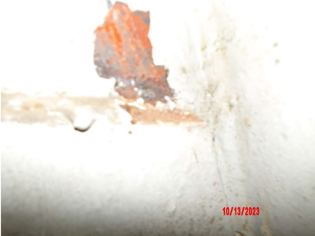
Photo 22- Span 23C, Cross Frames Poor Weld Quality to Girders
