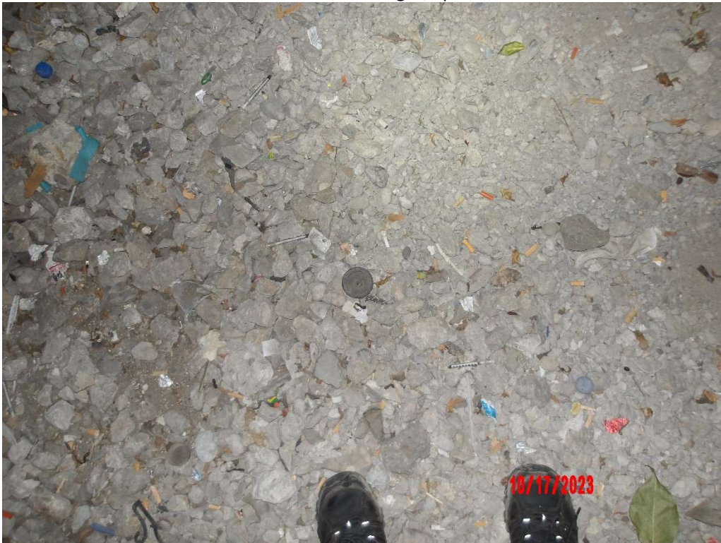
Photo 49- Span 29, Abutment C, Homeless Debris with Lots of Needles
