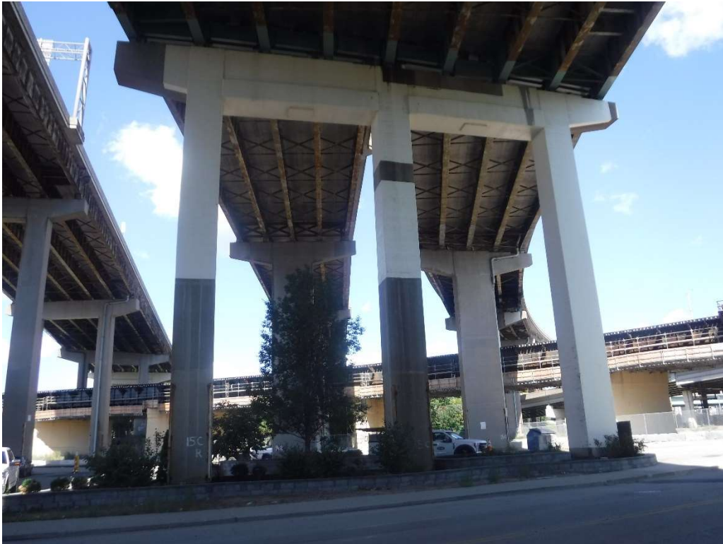
Photo 40- Pier 15 Back Face
