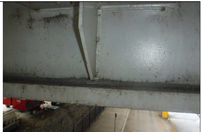
Photograph 13: Typical Example of Bottom of Knee Brace Weld Intersecting the Bottom Pier Cap Plate at Girder 4 North Side, Looking South.
