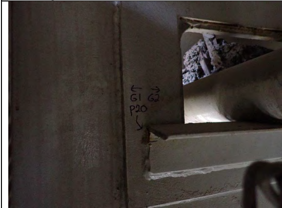
Photograph 21: Perspective View of 3/4 in. Crack to the Fillet Weld Between the Utility Support Angle and the Reinforcement Plate at the West End of the Angle, South Side of Cap Web Between Girders 1 and 2, Looking North.
