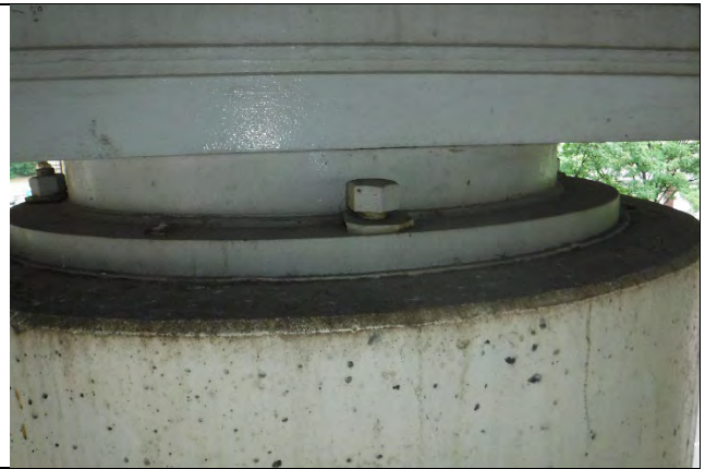
Photograph 15: Bearing Anchor Bolt Nut Not Fully Seated on the East Bearing with No Change, Looking North.
