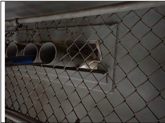
Photograph 19: Perspective View of 1 in. Crack to Fillet Weld Between Utility Support Angle and the Reinforcement Plate at the East End of the Angle, South Side of Cap Web Between Girders 2 and 3, Looking North.
