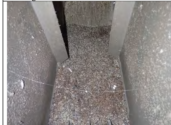
Photograph 11: View of the Bottom Flange Plate Between Diaphragms 7 and 8. Note Pigeon Debris Accumulating on Top of Plate, Looking East.
