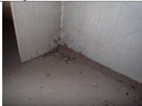
Photograph 26: Typical Example of Painted Over Section Loss at the Base of the Pier Cap Web Stiffeners and Web with No Change.
