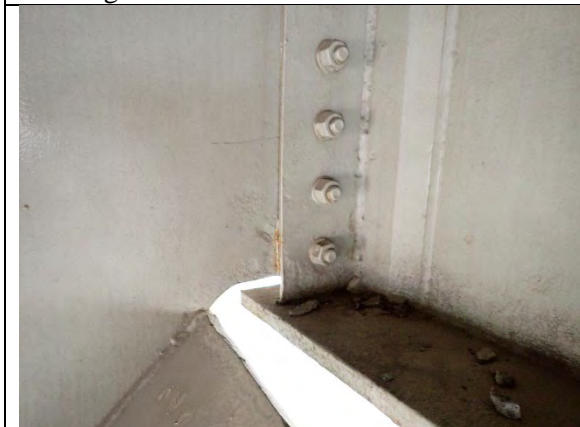
Photograph 25: Typical Example of Painted Over Section Loss at the Interface of the Hanger Bracket and the Pier Cap with No Change.
