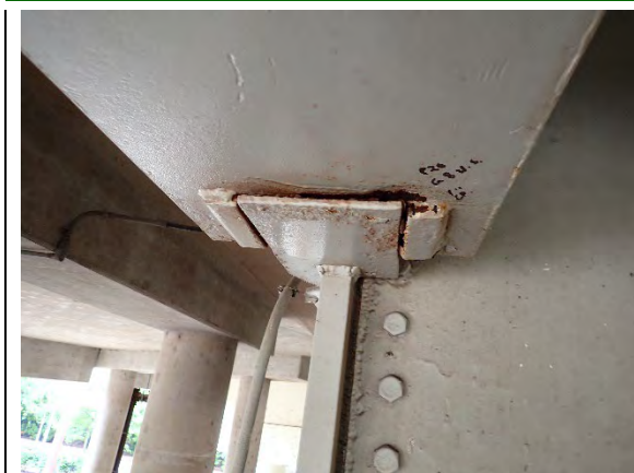
Photograph 23: Perspective View of 1 in. Crack in the Keeper Bar Weld at the North Side of Girder 8, Looking South
