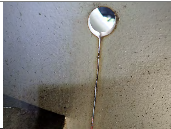
Photograph 10: Close-Up View of Typical Stress Relief Hole Retrofit at the Top Drilled Hole in the West Face of Diaphragm 1, Looking South.
