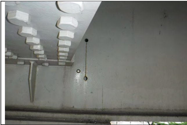
Photograph 14: View of Misdrilled Bolt Hole for Retrofit on South Side of Pier Cap in the East Face of Girder 1 with No Change, Looking North.
