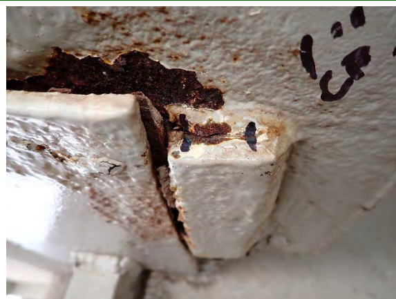
Photograph 24: Close Up View of 1 in. Crack in the Keeper Bar Weld at the North Side of Girder 8, Looking South
