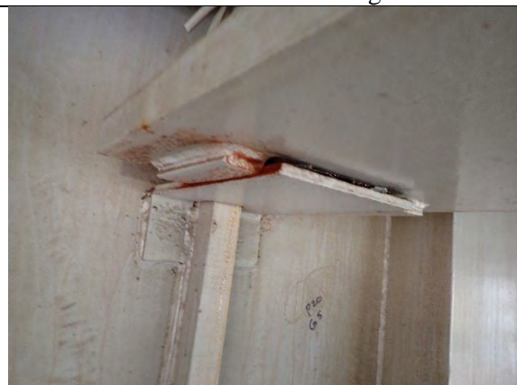
Photograph 28: Typical Example of Girder Bottom Flanges Rubbing Against the Keeper Plates with Up to 1/32 in. Wear on the Keeper Plates and No Change.
