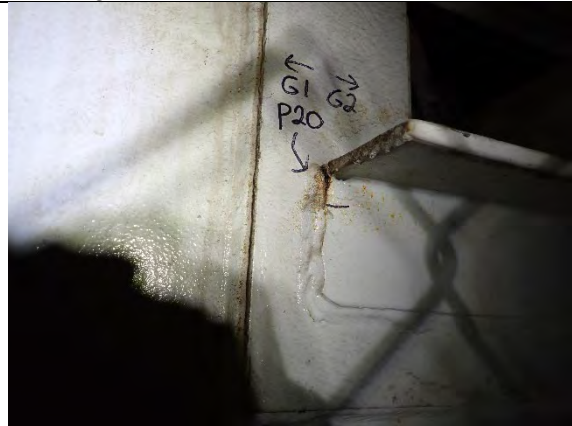
Photograph 22: Close Up View of 3/4 in. Crack to the Fillet Weld Between the Utility Support Angle and the Reinforcement Plate at the West End of the Angle, South Side of Cap Web Between Girders 1 and 2, Looking North.
