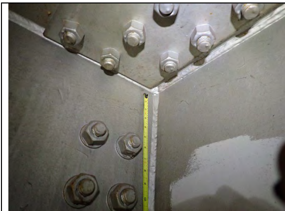
Photograph 7: View of West Face of Diaphragm 2 Under Tie Plate. Typical Triaxial Detail on Pier Cap Interior, Looking East.
