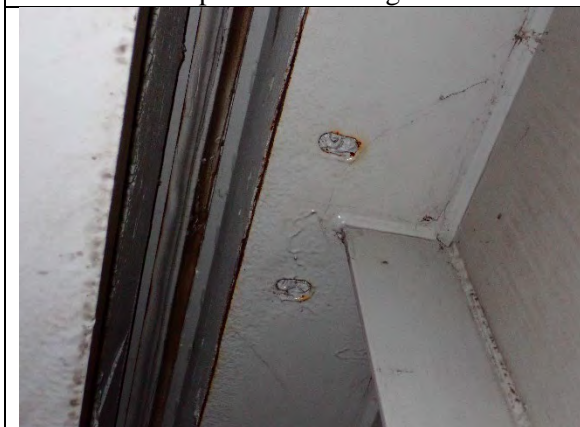
Photograph 27: Typical Example of Sheared/Missing Bolts on the Top Flange of the Pier Cap with No Change.
