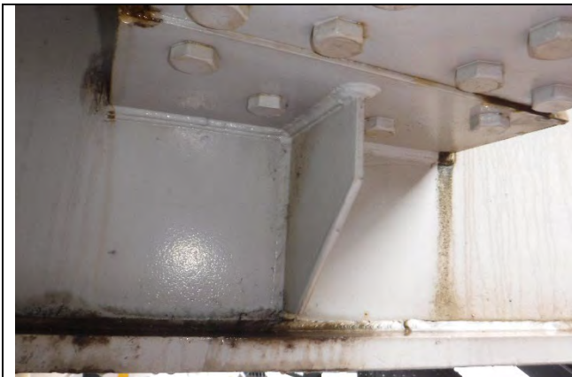
Photograph 12: Typical Example of Triaxial Welds at the Exterior of the Pier Cap. North face of the Cap at the Girder 1 Connection, Looking South.
