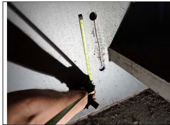
Photograph 9: Overall View of Typical Stress Relief Hole Retrofit in the East Face of Diaphragm 1, Looking South.
