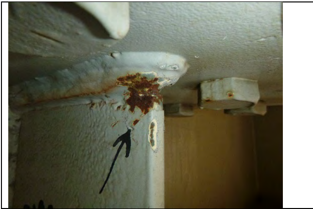
Photograph 18: 1/2 in. crack in the intersecting welds between the seat plate and the north side of the pier cap web plate at Girder 2, Looking Northeast.
