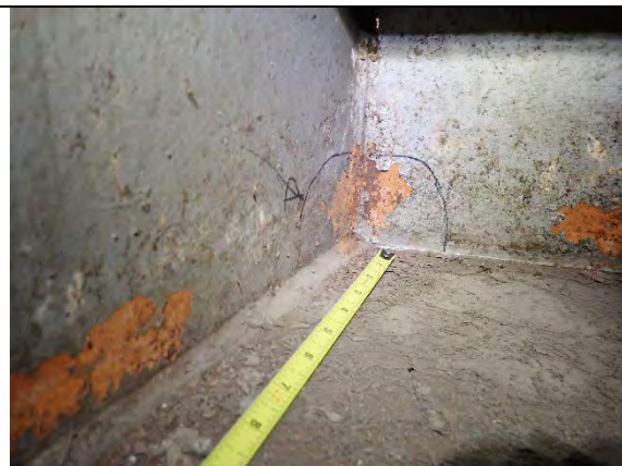
Photograph 8: View of West Face of Diaphragm 2 on Top of Tie Plate. Typical Triaxial Detail on Pier Cap Interior, Looking East.
