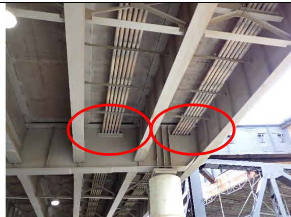
Photograph 17: View of West End of Pier 19, North Face. Note Cut Out Portion of Cap Web for Conduit. No Change.
