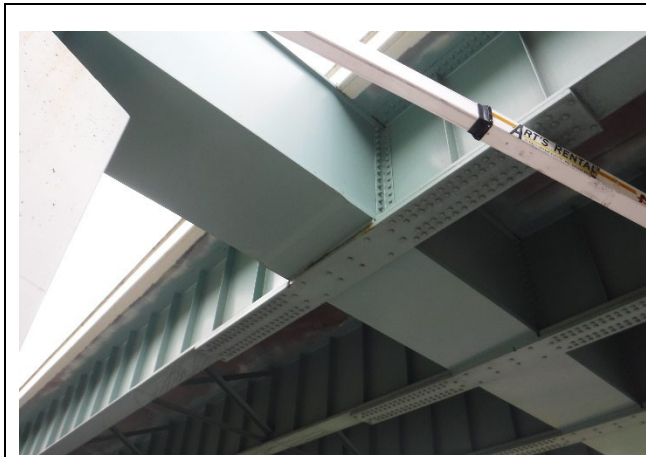
Photograph 3: General Underview of Pier Cap 1. Note Tie Plates, Bolted Clip Angles, and Overall Steel Configuration, Looking Northeast.
