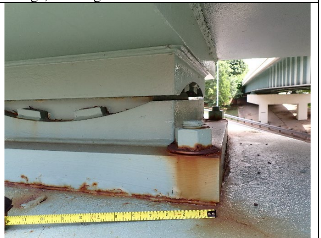
Photograph 12 – View of the Southeast Corner of the West Bearing. Note Typical Corrosion on the Masonry Plate and Anchor Bolts/Nuts, Looking North.
