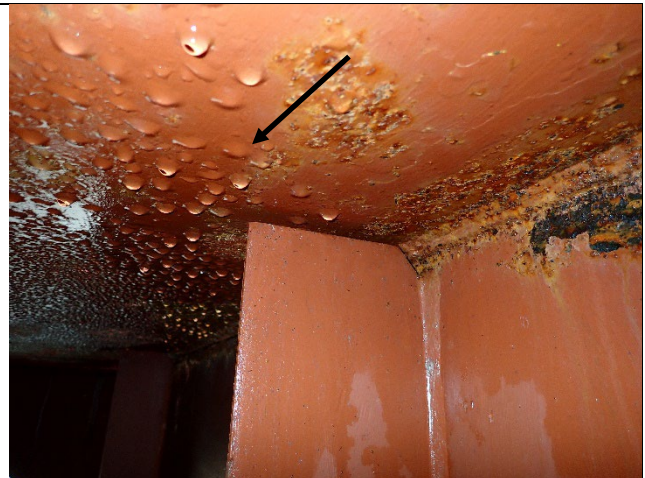
Photograph 4: View of North Web Plate Near West End Between Bearing Stiffeners and Diaphragm A. Note General Example of Condensation Present on Top Plate Due to Humidity, Looking Northwest.
