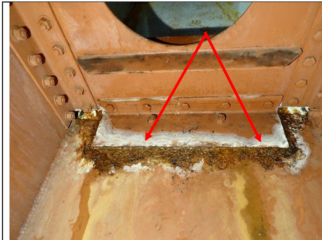
Photograph 7 – View of the Connection Angle Between the Bottom of the West Face of Diaphragm F and the Cap Bottom Plate. Note Active Corrosion Developing But No Pack Rust Present, Looking East.
