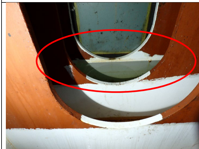
Photograph 5: View of Water Ponding Between the Bearing Stiffeners at the East End. Note The Easternmost Portion Was Completely Filled, Spilling Over to the Portion West of This, Looking East.
