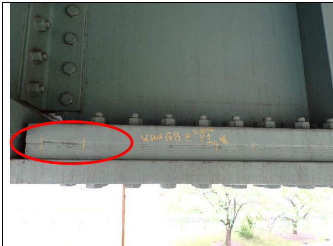
Photograph 9 – View of the West Face of the Bottom Flange of Girder B, South Side of the Pier Cap. Note No Change to the Tack Welds on the Bottom Tie Plate, Looking East.
