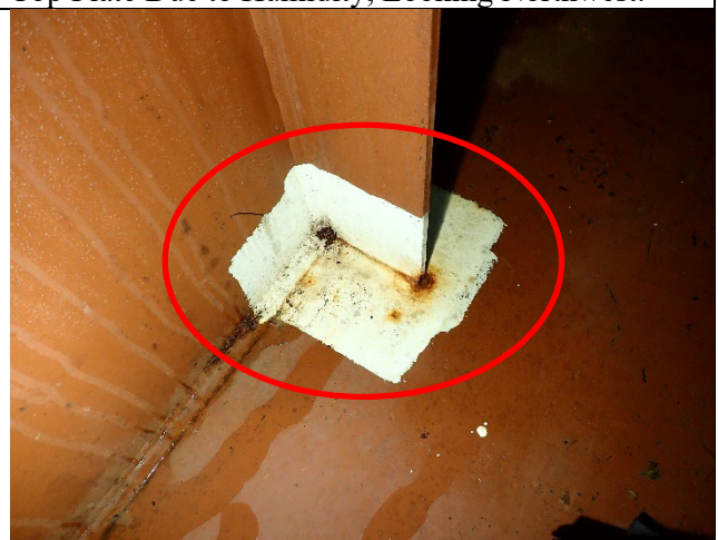
Photograph 6: View of the North Web Plate Between the West Hatch and Diaphragm A at the Base of the Stiffener. Note the Typical Example of Triaxial Weld at Base of Stiffener, Looking Northeast.
