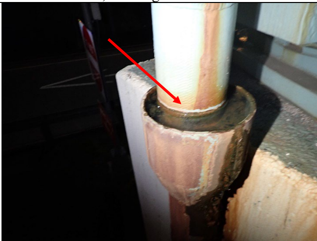
Photograph 11 – View of the Downspout on the North Side of the East Column. Note Downspout Was Still Clogged. No Change, Looking Southeast.
