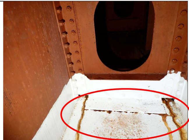
Photograph 8 – Typical Example of Lower Cap Interior With Recent Painting. Note Blistering Corrosion Developing at Isolated Areas on the Bottom Plate. The East Face of Diaphragm F Shown, Looking West.
