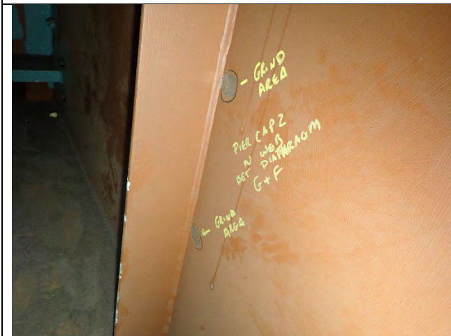
Photograph 6: General Example of Tack Weld Ground Down With Exposed Steel, North Cap Plate East of First Stiffener West of Diaphragm G Shown, Looking North.
