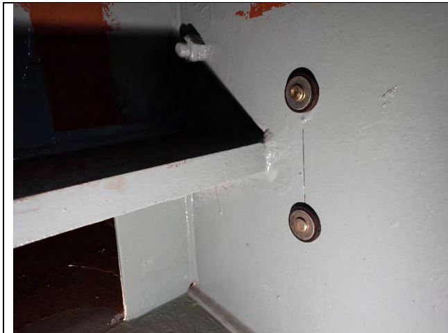
Photograph 21: View of Typical Stress Relief Retrofit. Diaphragm D North Cap Web West Face Shown, Looking Southeast.
