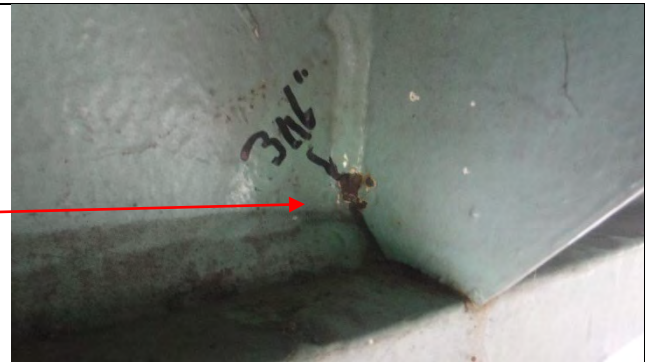
Photograph 26: Close Up View of 3/16 in. Long Crack in Vertical Weld For Knee Brace, Girder B at South Web Plate, Looking Northeast.
