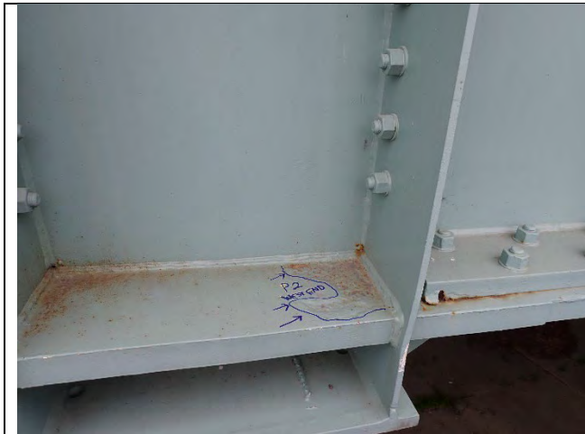
Photograph 16: View of 1/16 in. Deep Painted over Pitting On Tie Plate At West Side of Girder A, South Side of Pier, Looking East.
