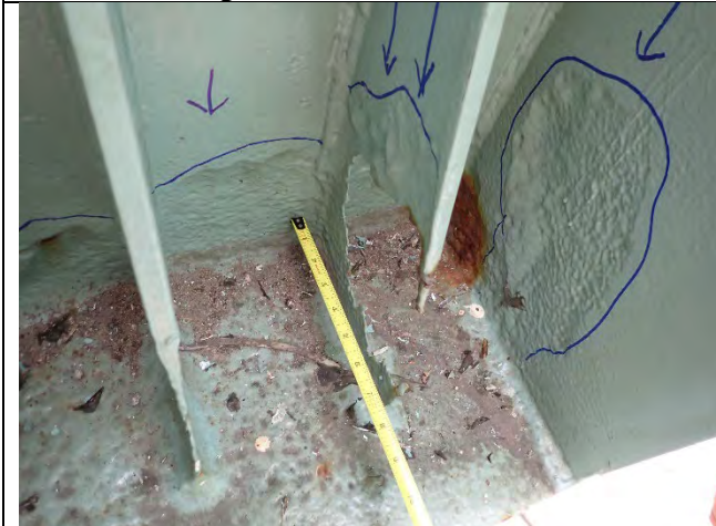
Photograph 29: View of Corrosion Hole at Base of North Knee Brace at East End of Cap, Looking West.
