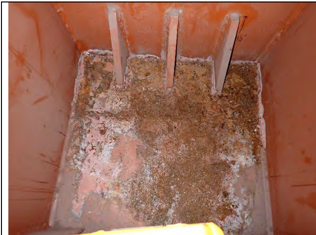
Photograph 32: View of Laminating Corrosion Present Just West of West Bearing on Bottom Plate, Looking West.
