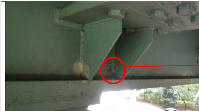
Photograph 25: Perspective View of 3/16 in. Long Crack in Vertical Weld For Knee Brace, Girder B at South Web Plate, Looking Northeast.
