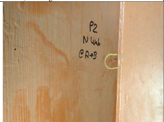
Photograph 7: General Example of Tack Weld Not Removed, North Plate Between Diaphragm A and B Shown, Looking Northeast.
