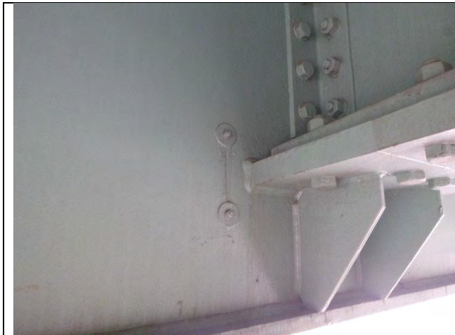
Photograph 37: View of Typical Stress Relief Retrofit. South Web Plate West Face of Girder D Shown, Looking Northeast.
