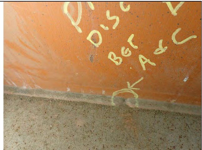
Photograph 33: View of Discontinuity For Fillet Weld Between North Cap Web and Cap Bottom Flange Between the Girders A and C Diaphragm, Looking North.
