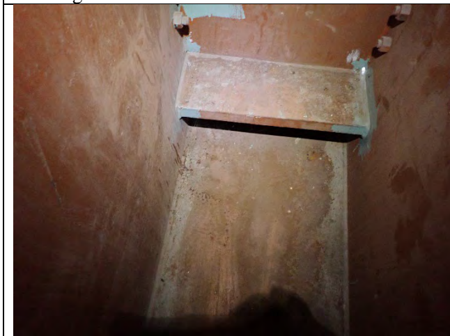
Photograph 10: View of Active Corrosion and Pitting over the West Bearing, Looking West.
