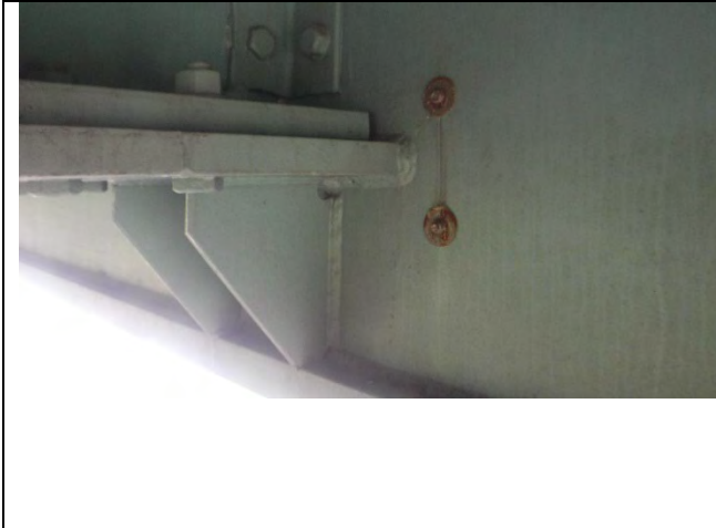
Photograph 27: View of Typical Stress Relief Retrofit. Diaphragm F South Cap Web East Face Shown, Looking Northwest.
