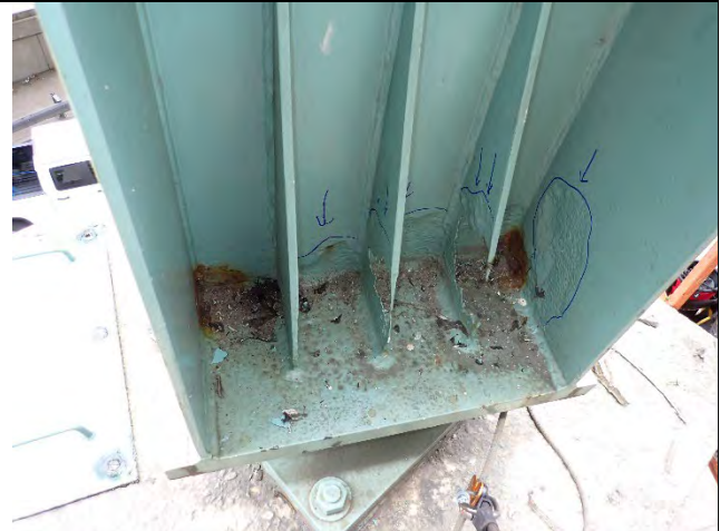
Photograph 28: Overall View of Painted over Pitting and Corrosion Holes at East End of Pier Cap.
