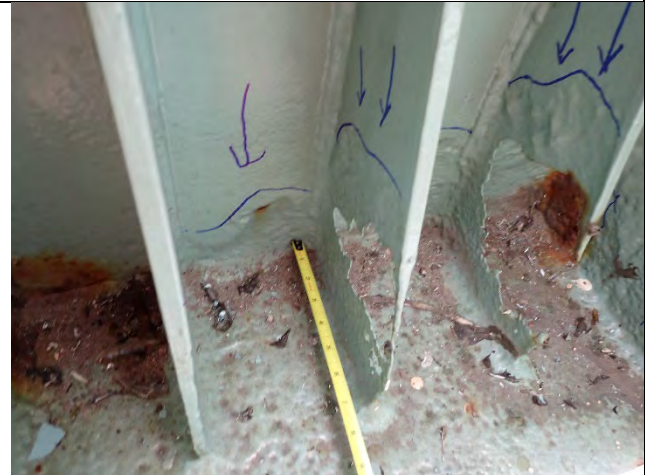
Photograph 30: View of Corrosion Hole at Base of Center Knee Brace at East End of Cap, Looking West.
