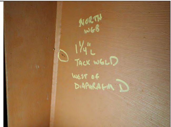
Photograph 22: View of Tack Weld Present on North Cap Web Plate, West of Diaphragm D. No Change, Looking Northwest.
