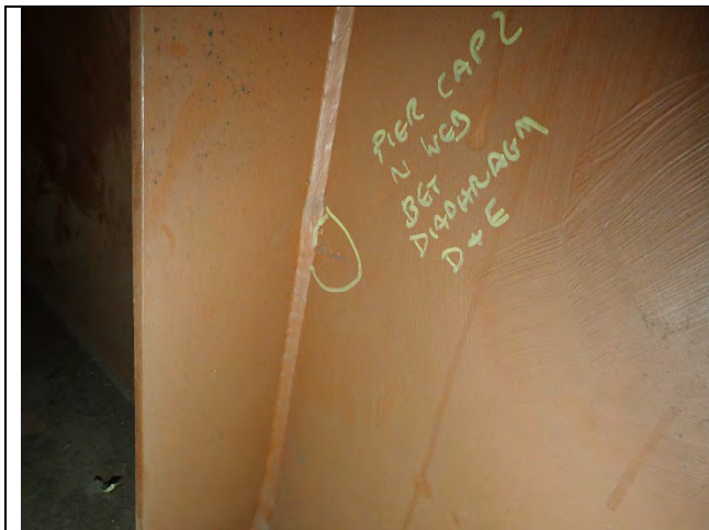
Photograph 8: General Example of Tack Weld Ground Down With Exposed Steel, North Plate East of Stiffener Between Diaphragms D and E Shown, Looking Northwest.
