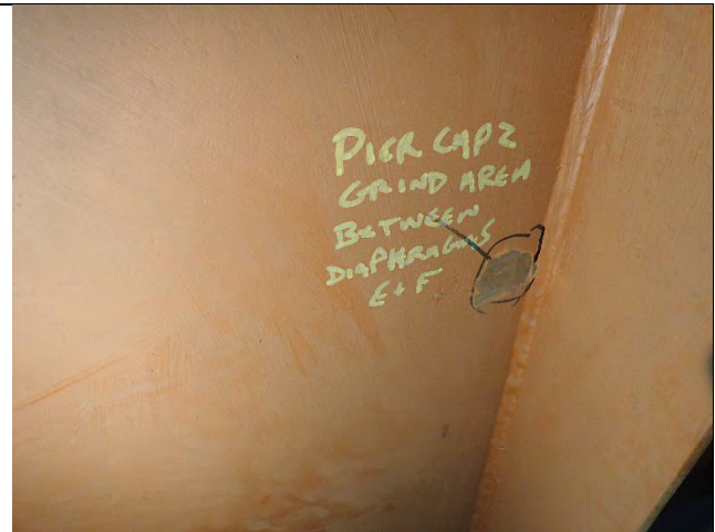
Photograph 5: General Example of Tack Weld Ground Down With Exposed Steel, North Cap Plate West of Stiffener Between Diaphragms E and F Shown, Looking North.
