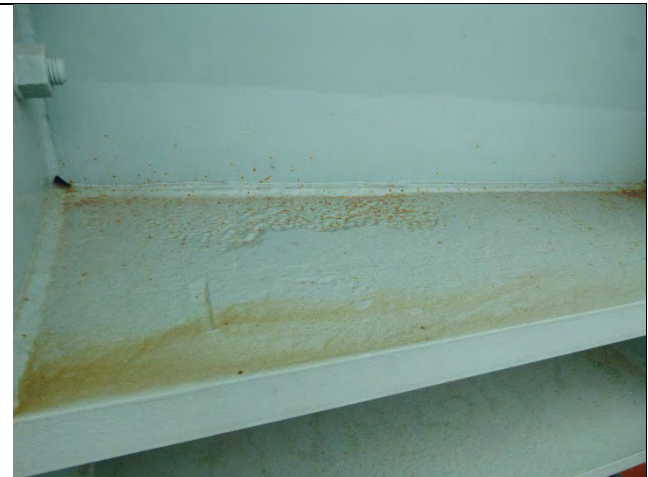
Photograph 38: View of Painted over Pitting To 1/16 in. Deep on Cap Bottom Flange Plate at the West End, Looking East.
