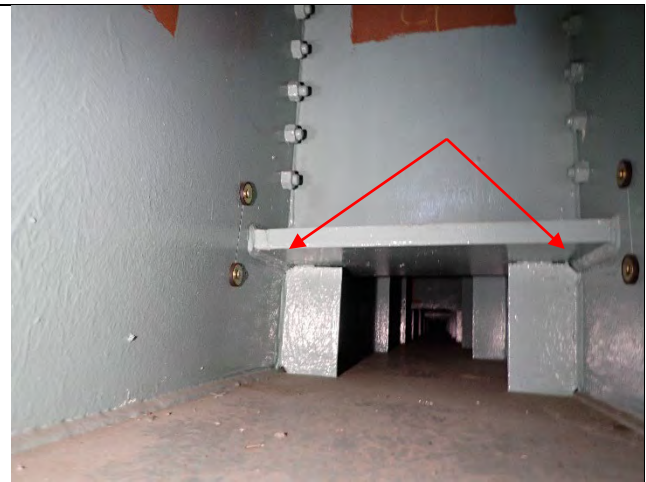
Photograph 20: View of East Face of Diaphragm G at Underside of Girder Tie Plates. Note Coped Corners of Lower Stiffener, Looking West.
