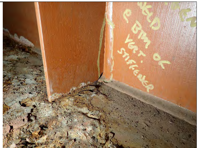
Photograph 35: View of Divergent Weld Located on the South Web Plate, First Stiffener West of West Bearing. Looking Southeast, No Change.
