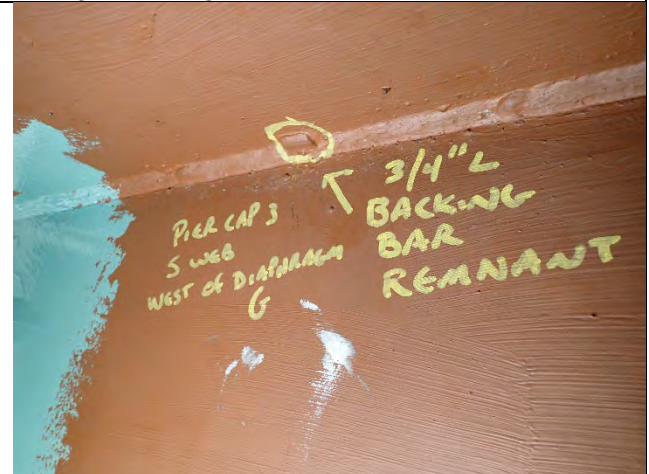
Photograph 24: View Backer Bar Remnant at South Cap Plate Top Weld, Between Diaphragm G and First Stiffener to the West, Looking South.
