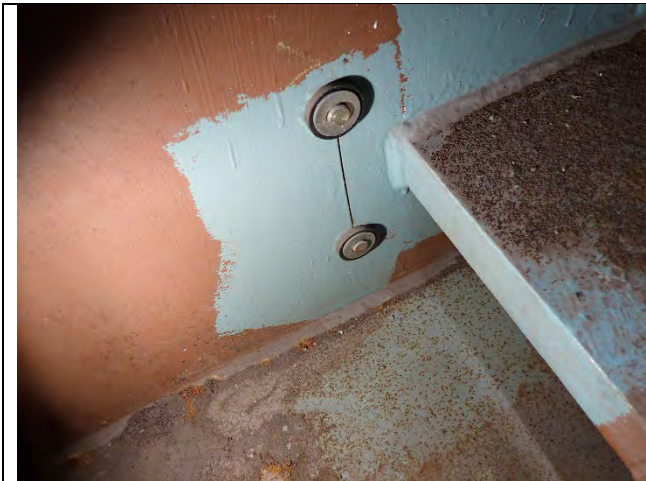
Photograph 4: View of Typical Retrofit At Internal Diaphragm. West Side of Diaphragm B Shown, Looking South.
