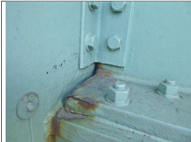
Photograph 39: View of Painted Over Pitting to 3/16 in. Deep On North Cap Web Behind Girder G Bottom Flange, Looking Southwest.
