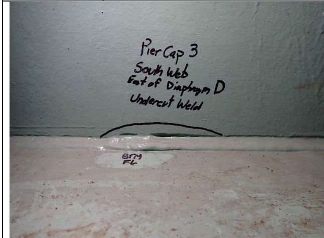
Photograph 23: View of Undercut Along South Cap Web Plate Bottom Weld, West of Diaphragm E, Looking South.
