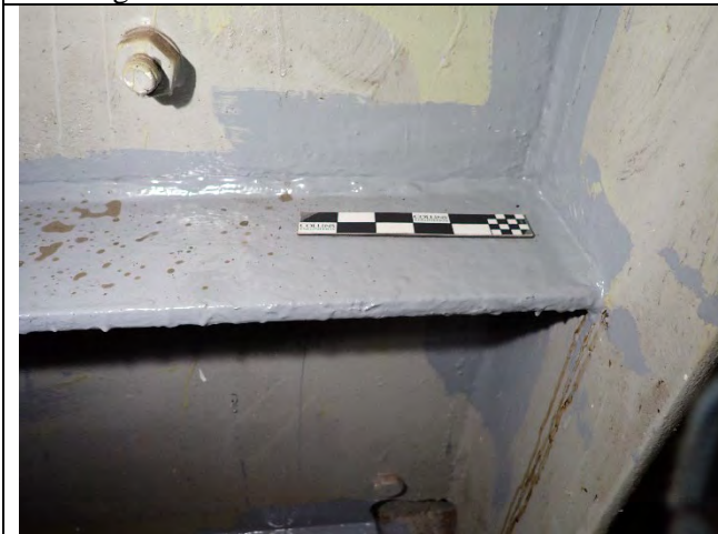
Photograph 7 – General Example of Intersecting Welds For Cap Web Plate Stiffeners Near Water Line. Looking east.
