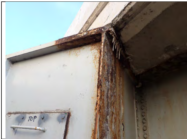
Photograph 12 – View of Laminating Corrosion on the South End of the Cap, East Side. Looking North.
