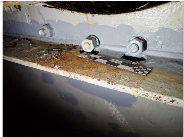
Photograph 6 – General Example of Holes Cut Through Fillet Welds of Horizontal Cap Web Stiffeners Below Water Line at Cap Web Plate. Looking West.
