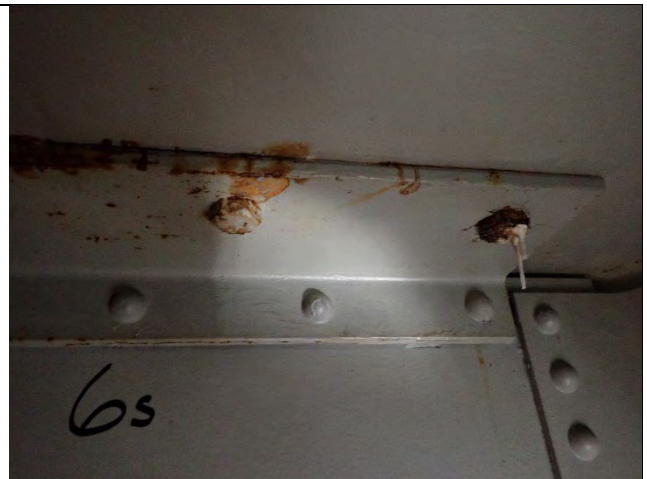
Photograph 4 – Typical Corrosion Through Clip Angle at Cap Top Flange Plate. Diaphragm 6 South Side Shown. Looking North.
