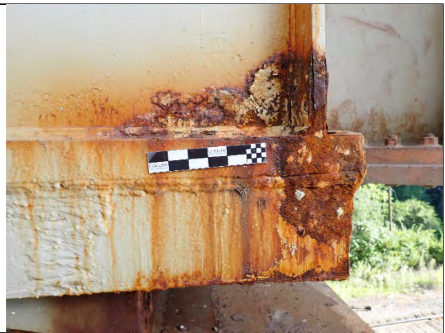
Photograph 13 – View of Laminating Corrosion on the South End of the Cap, Lower East Corner, With Isolated Pits to 1/8 in. Deep. Looking North.
