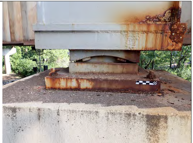
Photograph 17 – View of the South Bearing, Note Active Corrosion Continues, Heaviest On Masonry Plate. Looking North.
