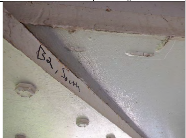
Photograph 15 – View of 3 Tack Welds Present on the West Side of the Cap Bottom Flange Between Girders 2 and 3. Looking East.
