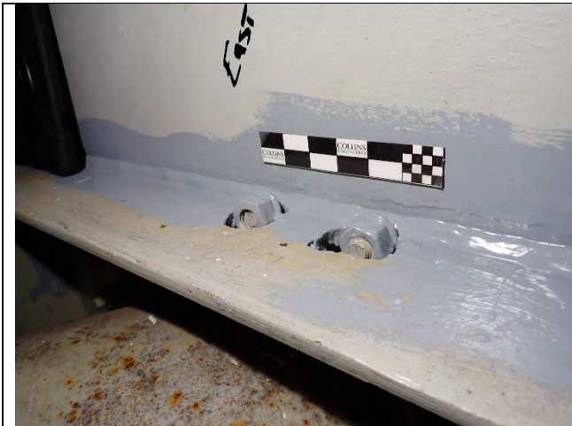
Photograph 5 – General Example of Holes Cut Through Fillet Welds of Horizontal Cap Web Stiffeners Above Water Line at Cap Web Plate. Looking West.
