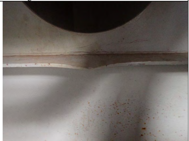
Photograph 8 – General Example of Bent Web Stiffener, Girder 6 North Side Shown. No Change. Looking South.
