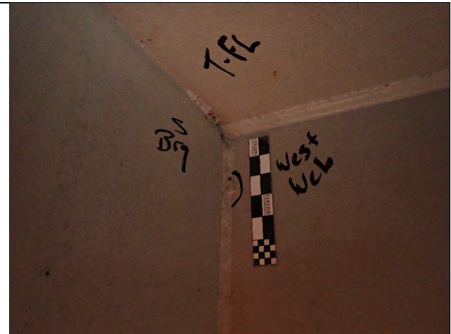
Photograph 10 – View of Tack Weld Located At the South Bearing Stiffener, West Cap Web Plate. Looking Southwest.
