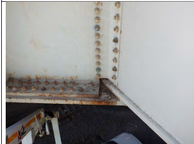
Photograph 14 – General Example of Active Corrosion on Cap With No Section Loss. South End West Face. Looking North.
