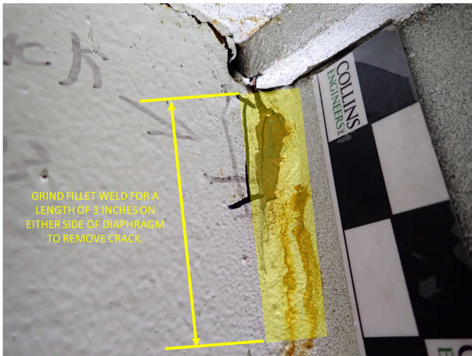
Figure 2 – Photograph of the observed crack illustrating recommended limits of grinding to remove the cracked portion of the fillet weld as well as a portion of the uncracked weld
