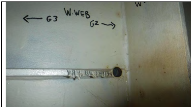
Photograph 38: Typical Longitudinal Stiffener Retrofit Detail.
