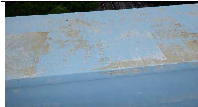
Photograph 8: Typical Fading Paint and Surface Corrosion at the South End of the Pier Cap, Looking West.
