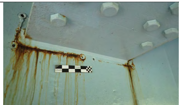
Photograph 34: Corrosion Was Beginning to Reactivate at Previously Painted Over Section Loss at Girder 5 and Pier Cap East Web Plate, Looking West.
