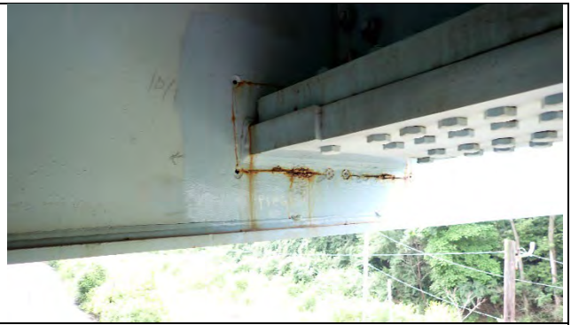
Photograph 50: Reactivated Corrosion at Girder 10, Looking Southeast. No Change Since the Last Inspection.
