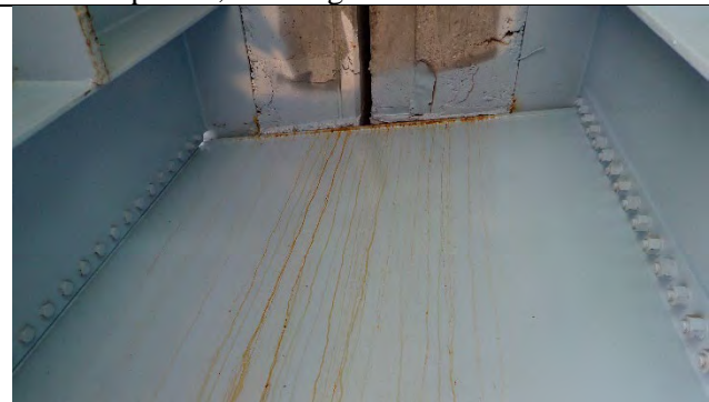
Photograph 59: View of Surface Corrosion on Top Flange Plate Edge and Rust Staining on Cap Web Plate, Looking West.
