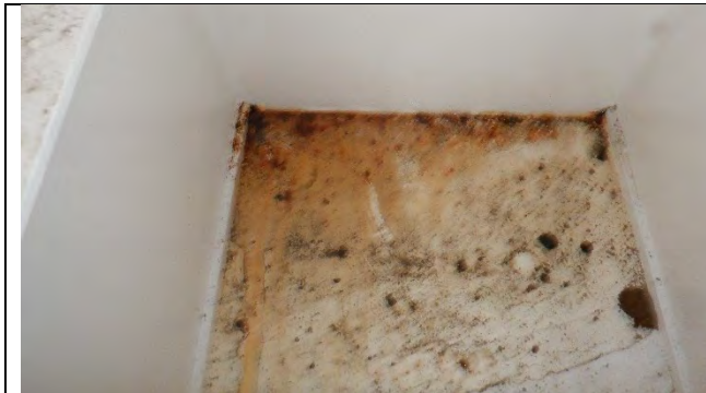
Photograph 15: Evidence of Ponding with Corrosion on the Bottom Flange on the South Side of Girder 5, Looking North.
