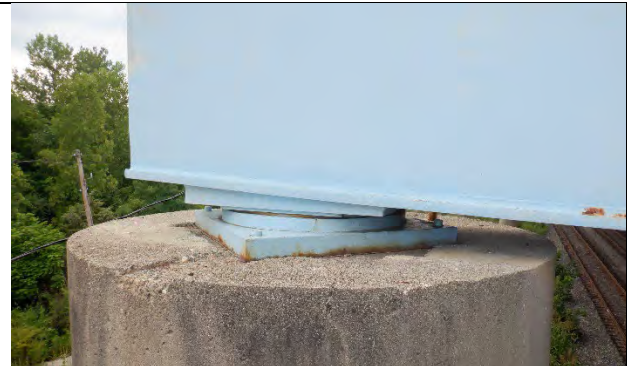
Photograph 43: South Bearing Masonry Plate Corrosion, Looking West.
