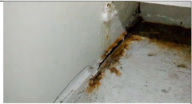
Photograph 46: Rust Staining from Retrofit Holes at Girder 10.
