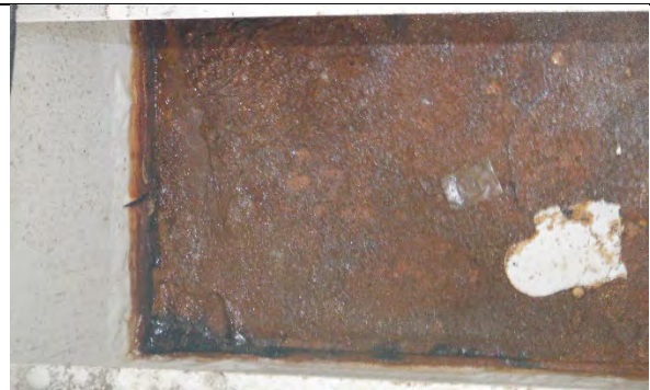
Photograph 31: Typical Ponding Water and Surface Corrosion on Bottom Flange.
