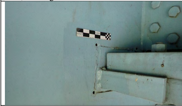
Photograph 51: No Change to 1/16 in. Bow/Indentation Previously Observed, Looking Northwest.
