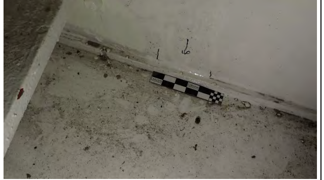
Photograph 56: Newly Observed 4.5 in. Fillet Weld Along the Lower Corner of Diaphragm 6, Looking East.
