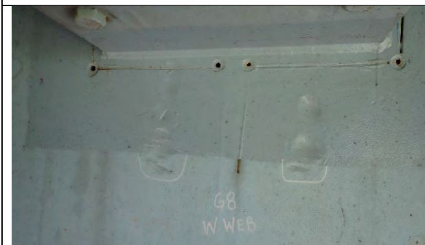
Photograph 35: Heavy Gouging on West Web Plate Below Girder 8 From Girder Knee Brace Removal, Looking East.
