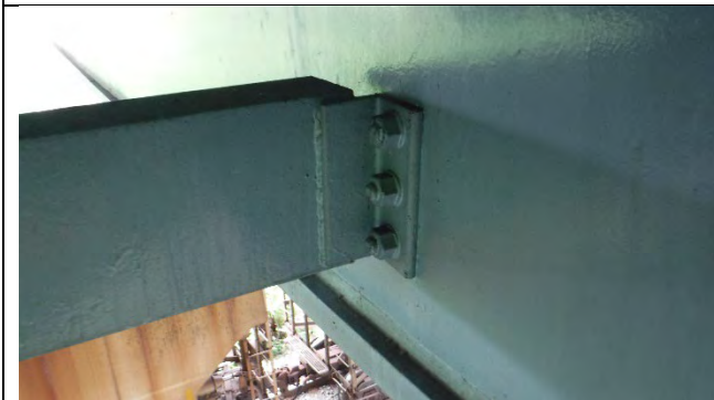
Photograph 25: Bolted Connection Between the Girder 6 Drain to the South Web Retrofit.
