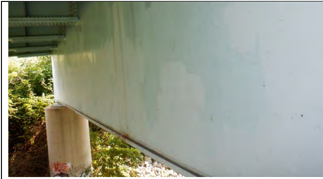
Photograph 42: Typical Pier 7 Paint Condition.
