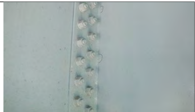
Photograph 9: Five 1 in. Tack Welds on the West Web at the South Face of Girder 9, Looking East.
