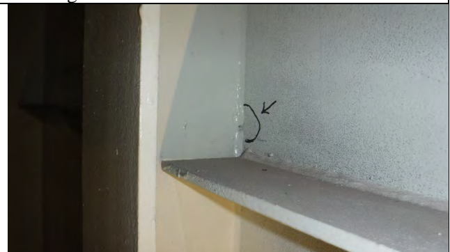
Photograph 41: 1.25 in. Discontinuity in the Transverse Stiffener Weld on West Web Between Girders 7 and 8, Looking East.
