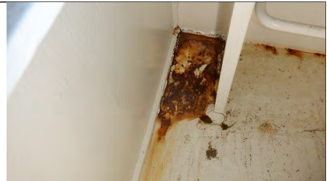
Photograph 16: Typical Corrosion on the South Side at the Bases of the Diaphragm, Looking North.
