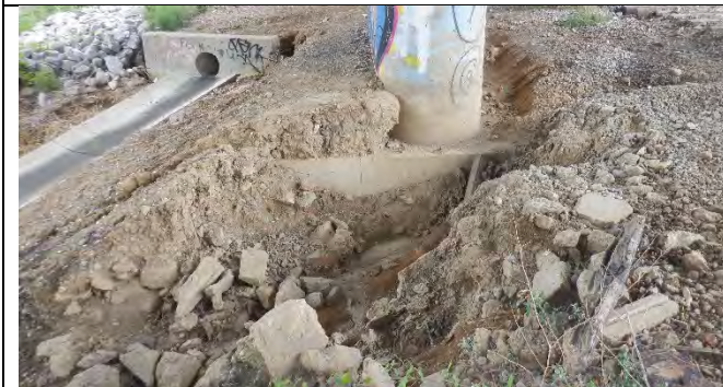
Photograph 12: Erosion at the Base of the East Column, Looking East.
