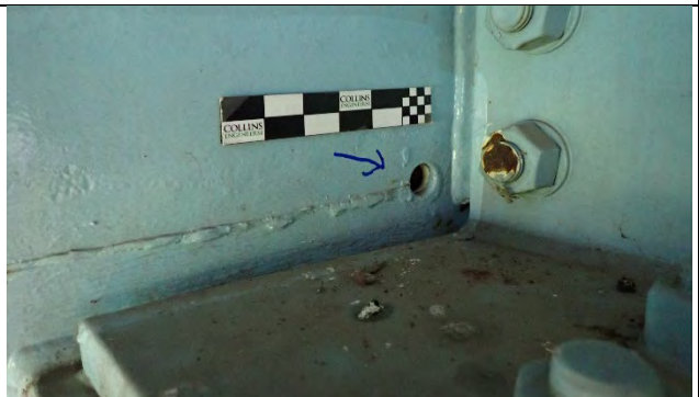
Photograph 60: Typical Example of Missing Expansion Plugs, Looking East.
