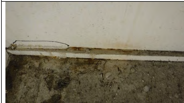
Photograph 40: Corrosion Has Reactivated Between Backer Bar and East Web Near Welds, Looking West.
