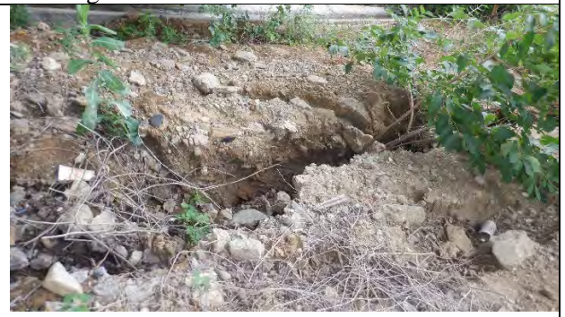
Photograph 13: Erosion at the Base of the North Column, Looking East.
