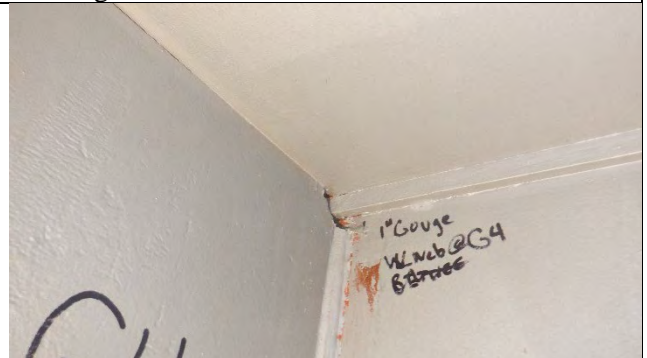
Photograph 22: 1 in. Gouge in the West Web on the North Side of Girder 4, Looking West.
