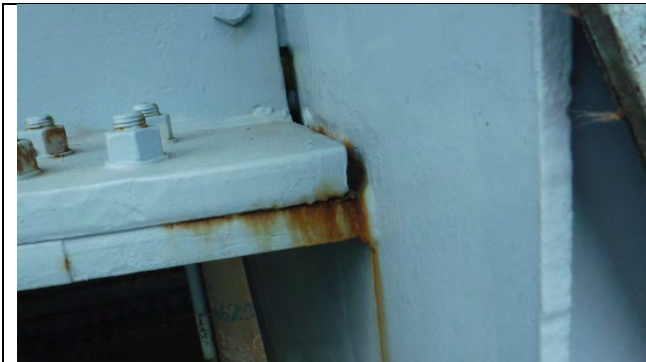
Photograph 23: Reactivated Corrosion at Previously Painted Over Section Loss on the East Web at Girder 1.
