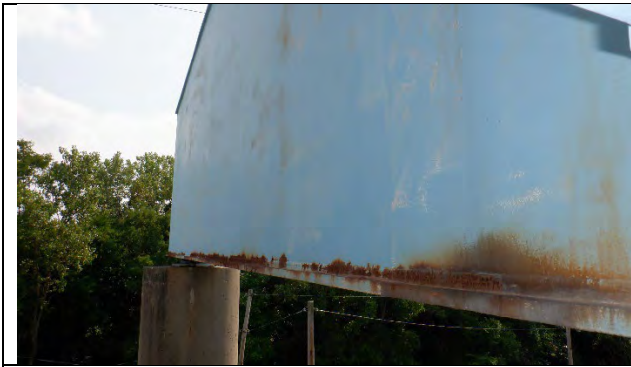
Photograph 49: Surface Corrosion with No Section Loss Along the Lower Corner of the Cap on the East Face, Looking Southwest.
