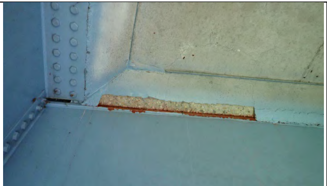
Photograph 58: No Change to Spall Along Haunch, Looking East.
