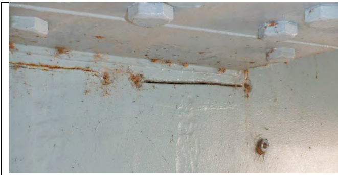
Photograph 10: Rust Staining on the East Web Retrofit at Girder 7, Looking Northwest.
