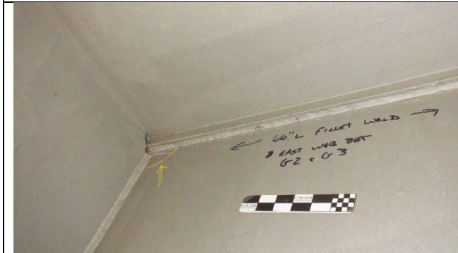
Photograph 21: 1.5 in. Gouge in the East Web on the South Side of Girder 2, Looking East.
