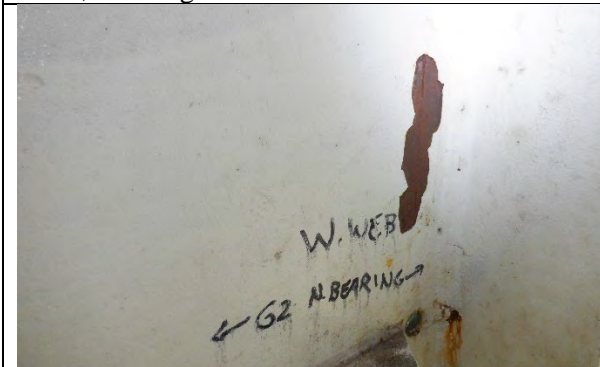
Photograph 32: Typical Paint Defect and Surface Corrosion Due to Missing Epoxy Sealant at Retrofit.
