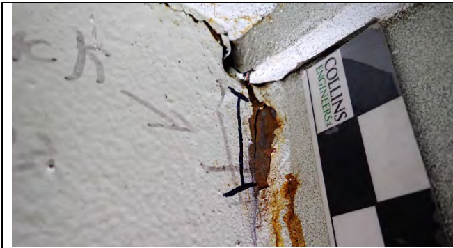
Photograph 30: View of 1.5 in. Weld Crack at the Top of the Fillet Weld for the Diaphragm to West Web Plate at Girder 6, North Side of Diaphragm. Close-Up View, Looking South.
