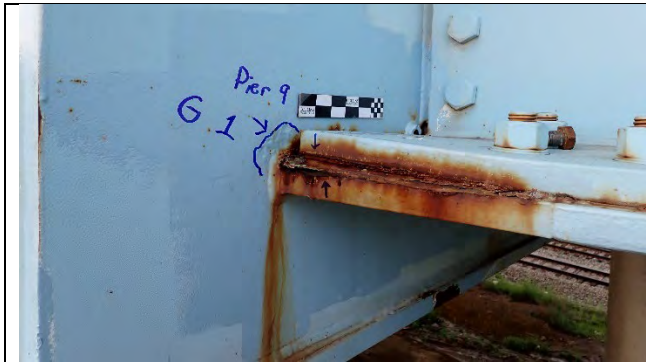
Photograph 57: Pack Rust Up To 1/2 in. Between Girder and Tie Plate and Painted Over Pitting to 1/16 in. on Cap Web, Looking Southeast.
