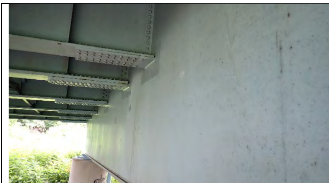
Photograph 33: Typical Condition of the Exterior of Pier 6 at the West Web Plate, Looking North.
