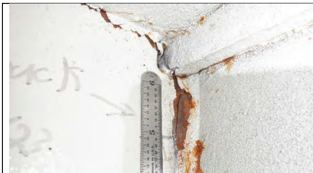
Photograph 28: View of 1.5 in. Weld Crack at the Top of the Fillet Weld for the Diaphragm to West Web Plate at Girder 6, North Side of Diaphragm. Perspective View, Looking South.
