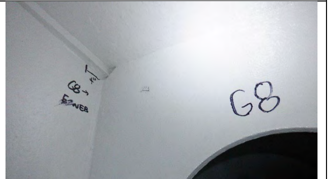
Photograph 49: Weld Extending Through Web Cope at Girder 8, Looking Southeast.
