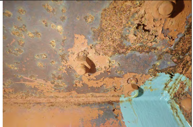
Photograph 63: Typical Example of Oversized Bolt Holes on Cap Top Flange Plate, Diaphragm M East Face Shown.
