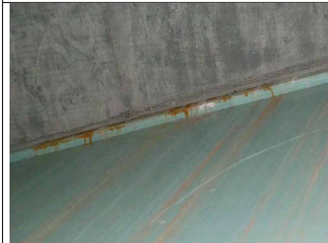
Photograph 36: View of the Typical Rust Staining on the South and North Web of the Cap.
