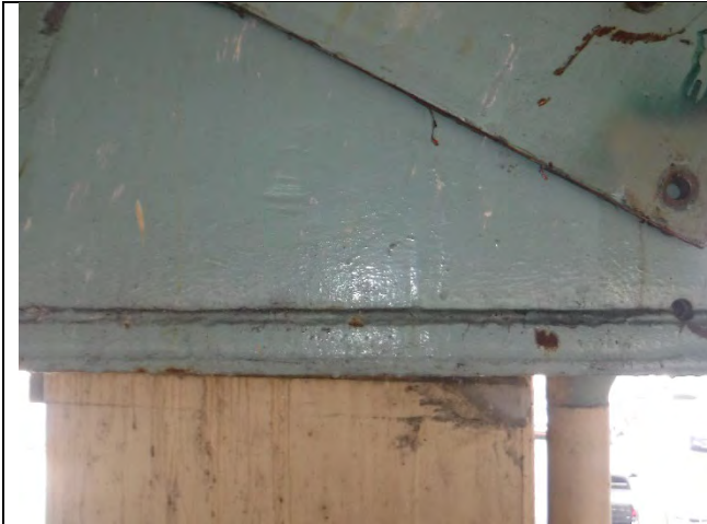
Photograph 28: View of the Retrofits Performed on the Exterior of the Pier 2W Cap.
