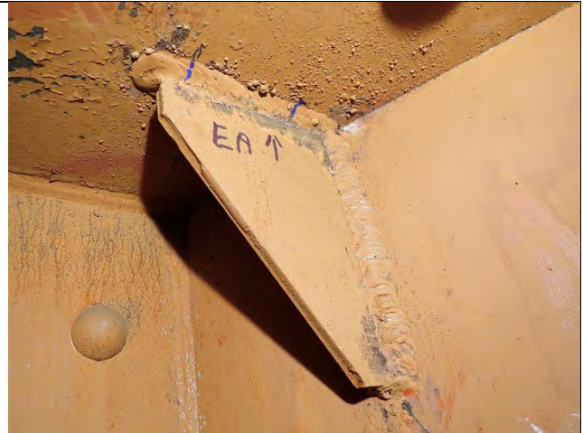
Photograph 42: Visual Crack Indication at Girder EA. Indication was Tested with Magnetic Particle and Determined to Not Be A Crack.
