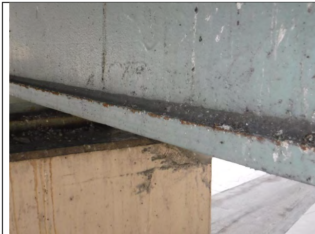
Photograph 26: View of the Minor Surface Corrosion Noted on the Bottom Flange of Pier Cap 2W.
