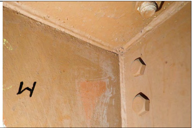
Photograph 23: Typical Example of Intersecting Welds Inside Pier Cap 2W.
