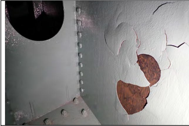
Photograph 13: Failed Paint and Active Corrosion on North Web Plate Between Girders M and N, Looking Northwest.
