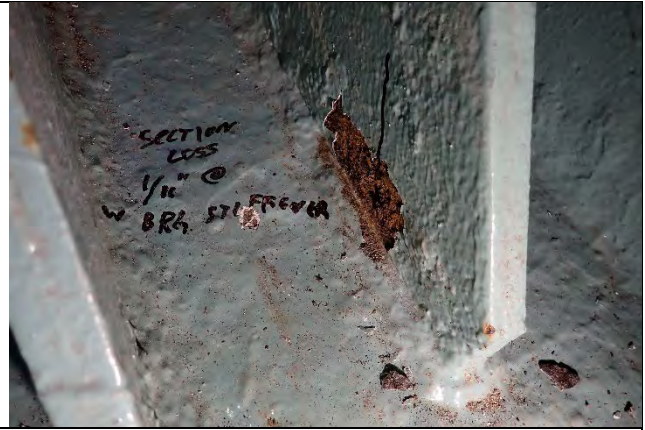
Photograph 14: View of Section Loss to 1/8 in. on Braces Near the East Bearing Stiffener, Looking West.
