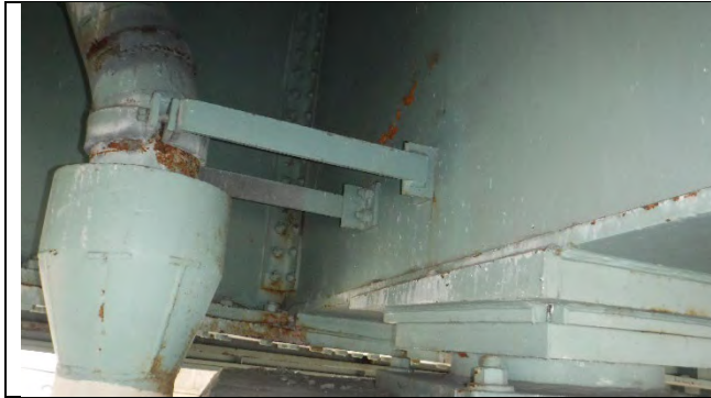
Photograph 19 – View of Bolted Connections that replaced Welded Connections for Drainage System. Looking Southeast.
