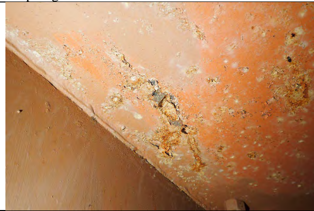
Photograph 24: General Example of Flaking Paint and Active Surface Corrosion along the Top Plate. Occurs Randomly but Consistently along the Plate.
