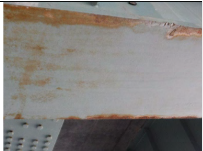
Photograph 27: View of the Minor Surface Corrosion Noted on the Bottom Flange of Pier Cap 2W.
