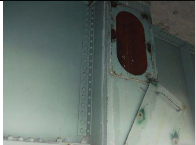
Photograph 29: View of the Retrofits Performed on the Exterior of the Pier 2W Cap.
