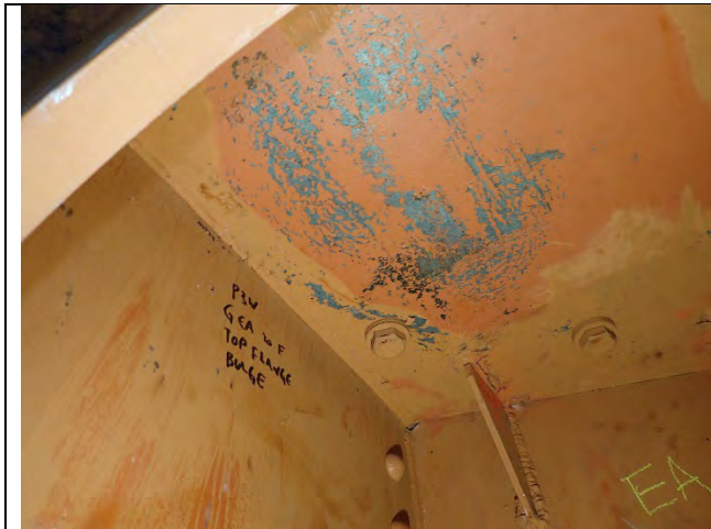
Photograph 45: View of Large Bulge in the Top Flange between Girder EA to F with Loss of Paint.
