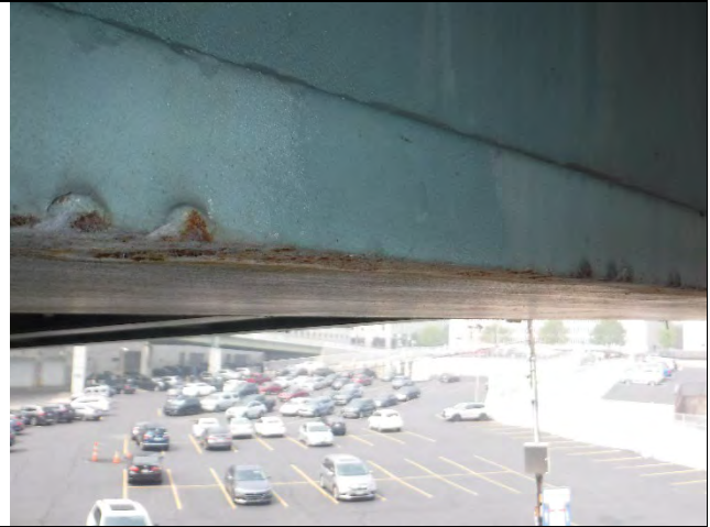
Photograph 31: View of the Gouges at the North Edge of the Bottom Flange over the Length of the Pier Cap, most of which are near Girder D.
