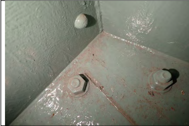
Photograph 15: Typical Example of Intersection Welds, Lower North Web Plate West side of Diaphragm J Shown Looking Northeast.
