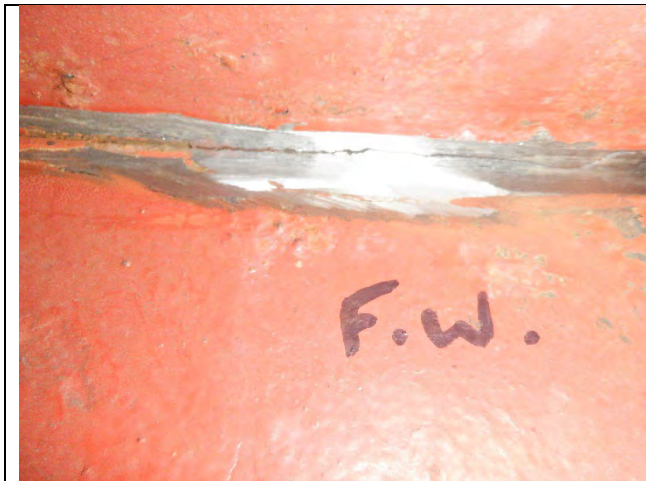
Photograph 56: Example of Ground and Removed Intermittent Tack Welds Between the Top Flange and Bearing Stiffeners at Both West Bearing Stiffeners.
