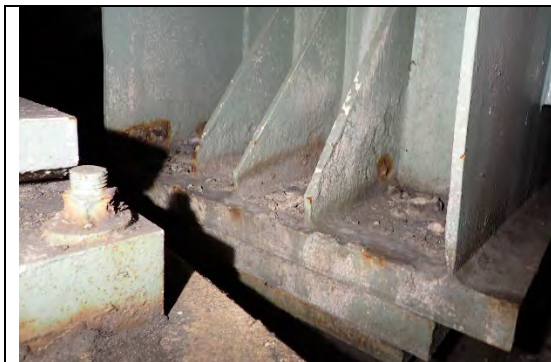
Photograph 65: Example of Painted over Pitting to 1/16 in. Deep on West Bearing Stiffeners.
