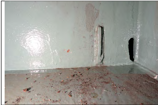
Photograph 22: Typical Example of Remnants of Knee Brace Connections Removed. East Face of Diaphragm E Shown.
