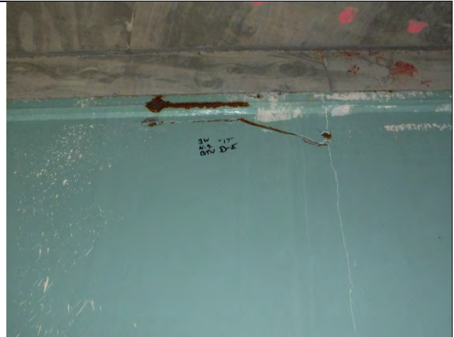
Photograph 52: View of the Impact Gouge Located on the North Side of the Cap in the Web and Flange between Girders D and E.
