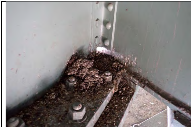
Photograph 58: View of the Typical Pigeon Debris Near End of Girders, East Face of Girder E Shown.
