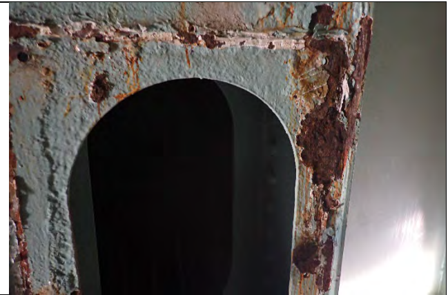
Photograph 18: View of East End Plate At Top of Hatch With Door Removed. Note Corrosion and Section Loss up to 1/8 in. Looking West.
