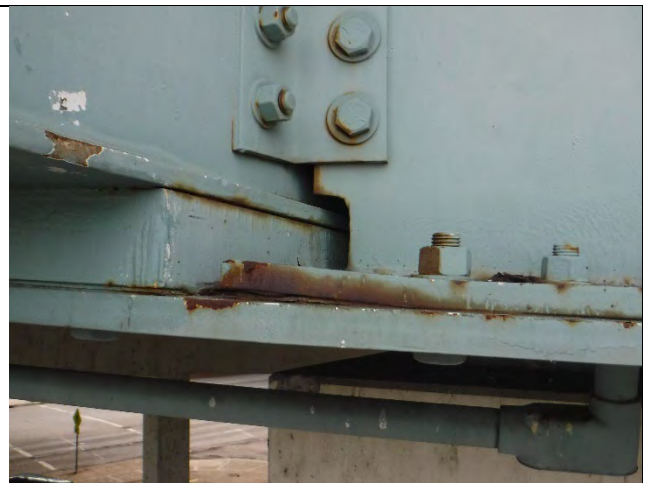
Photograph 50: View of the Pack Rust with Section Loss on the West Side of Girder A Between the Bottom Flange Plate and Tie Plate.
