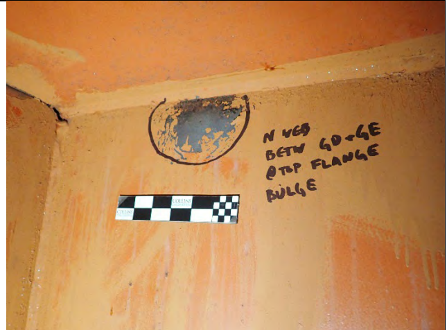
Photograph 44: Two minor bulges on a stiffener in the north web near the top flange between Girders D and E.
