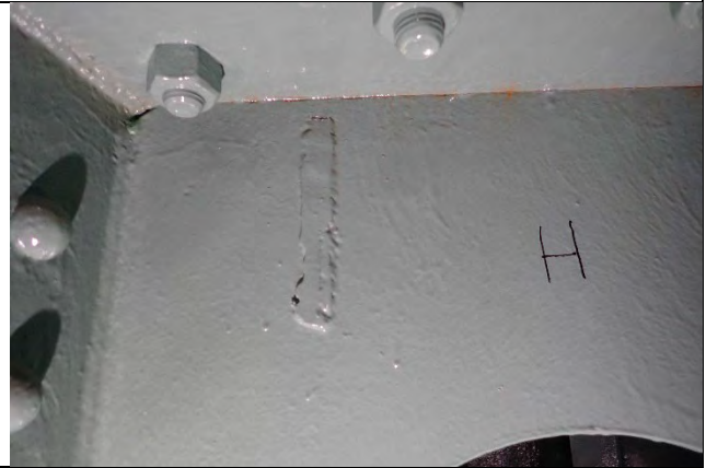
Photograph 16: Typical Example of Removed Knee Brace from Interior Diaphragm. Top of Diaphragm H shown. Looking West.
