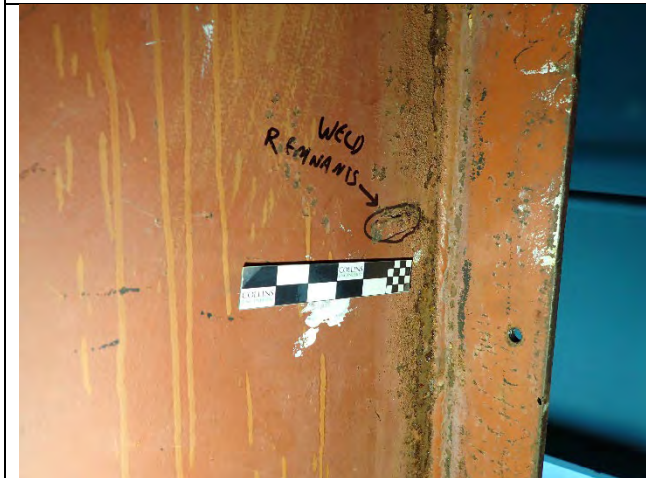
Photograph 47: Two Errant Weld Strikes Up to 2 in. Long Located on the North and South Web of the Cap Near the East Access Hatch.
