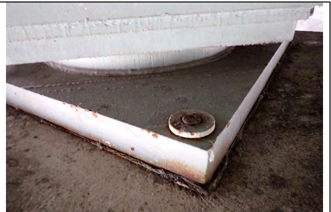
Photograph 11: Sheared Southeast Anchor Bolt at East Bearing, Looking Roadway Northeast.
