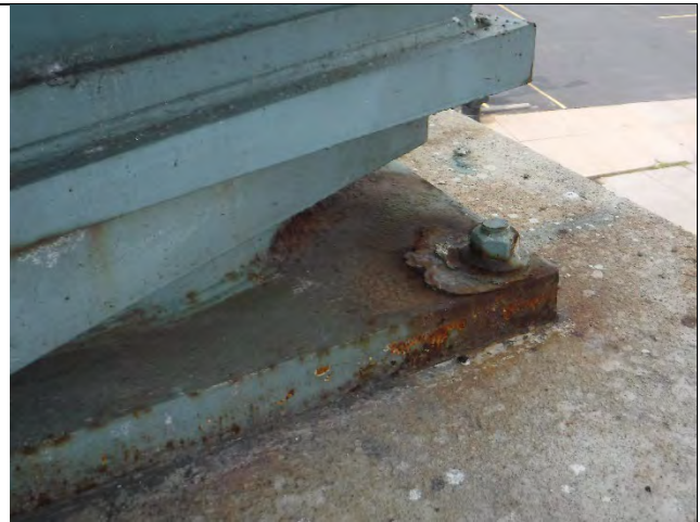
Photograph 39: View of the West Bearing with Moderate Surface Corrosion and Section Loss Around the Northwest Anchor Bolt.
