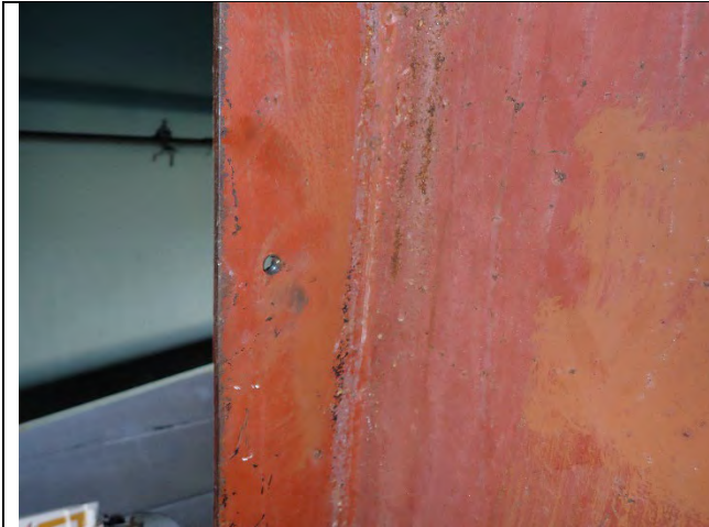
Photograph 41: Isolated Locations of Surface Corrosion Inside the Cap, Mostly at the Ends Near the Hatches.
