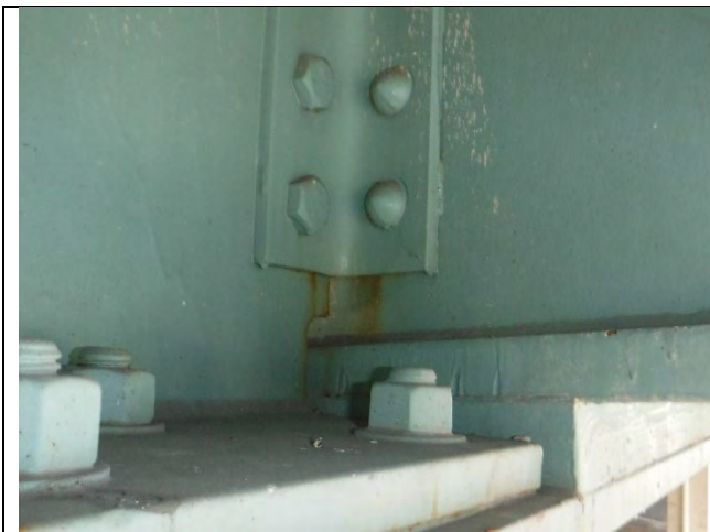
Photograph 49: View of the Remaining Tack Welds on the Bottom Flange at the West Edge of Girder B fill Plate, the West Edge of Girder E, and at the East Edge of the Girder EA Fill Plates.
