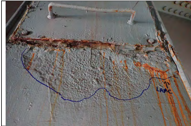
Photograph 17: View of East End Plate Below Hatch. Note Reactivated Corrosion and Section Loss up to 1/8 in. Looking West.
