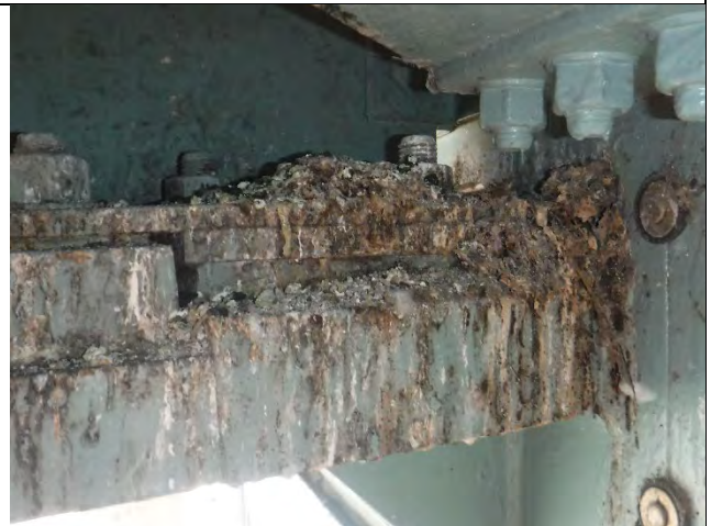
Photograph 35: View of the Pigeon Nests and Construction Debris was Observed on the South Web and Girder Lower Flanges.
