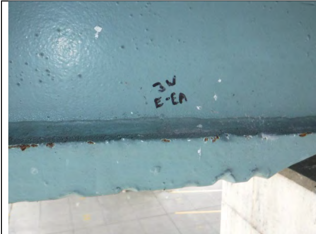
Photograph 51: View of Gouges on the South Edge of the Bottom Flange between Girders E and EA.
