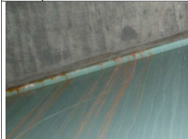
Photograph 34: View of the Moderate to Heavy Fretting Rust on the North and South Faces of the Cap along the Top Flange to Deck Interface Between Girders C and D.
