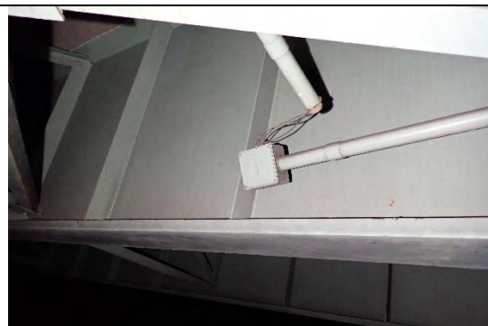
Photograph 66: No Change to Damaged Conduit on West Face of Girder N, North of the Cap.
