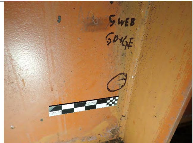
Photograph 46: View of Gouges at Stiffener Diaphragms. These Gouges are not a Structural Concern. South Web Between Girders D and E.
