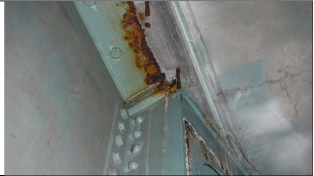
Photograph 20 – View of Active Corrosion on the Girder Top Flange and Cap Top Flange Plate East of Girder N. Looking North.
