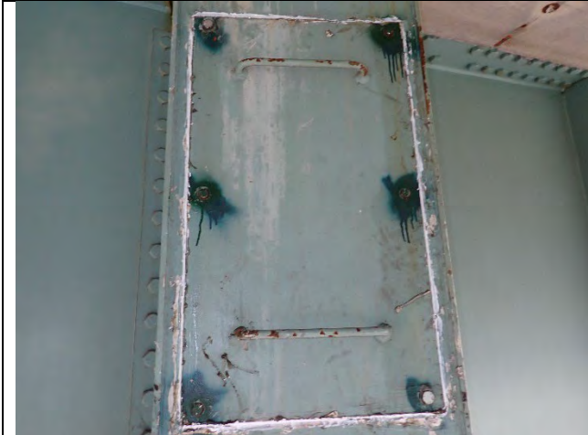
Photograph 43: Two out of six bolts were previously missing on the east access hatch but have been replaced. The open holes were caulked and sealed to prevent moisture infiltration.
