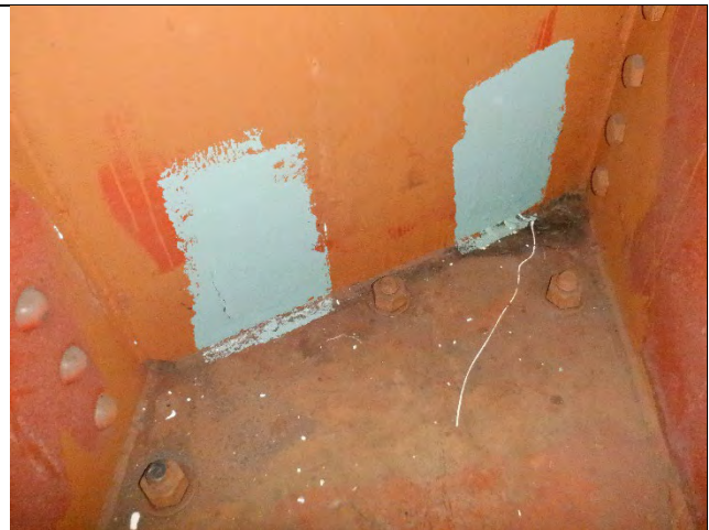
Photograph 57: View of Removed Welded Knee Braces on Cap Interior, and Intersecting Welds Between Cap Web Stiffeners, Bottom Flange, and Web Plates. Girder D Shown.
