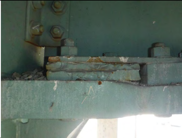
Photograph 30: View of the Deformation and Minor Section Loss Exhibited on Plates between the Tie Plate and Girder on the East Side of Girder F on the North Side of the Web.
