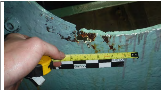
Photograph 8: View of 100% Section Loss Measuring 1 1/2 in. in Length at East (Compass South) Hatch Opening. Looking West.
