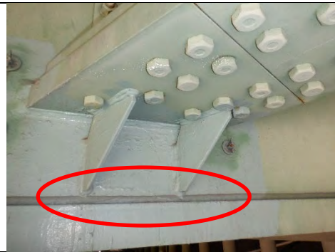
Photograph 11: Typical Example of Girder Knee Brace Welds Intersecting the Cap Web To Cap Bottom Flange Weld. Looking North.
