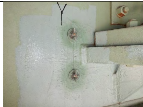
Photograph 9: Typical Example of Drilled Hole and Sawcut Retrofit. South Cap Web West Side of Girder Y Shown. Looking North.
