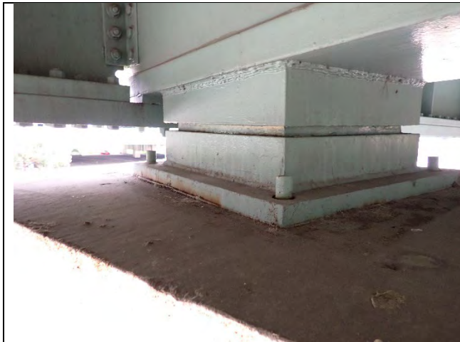
Photograph 22 (left): View of the Typical Missing Nut at the Bearing.
