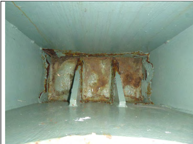
Photograph 24: Laminating Corrosion at the Ends of the Interior of the Pier Cap Has Reactivated.
