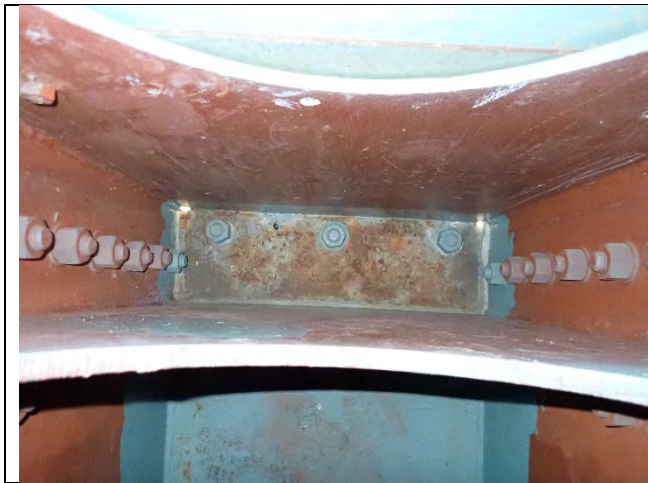
Photograph 16: Example of Corrosion Reactivating on the Bottom Flange Plate, West End Shown.
