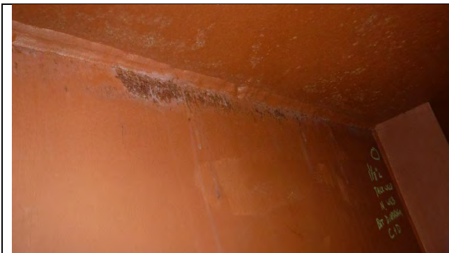
Photograph 4: Typical Example of Corrosion on Web Plates, North Web Between Diaphragms C and D Shown, Looking North.
