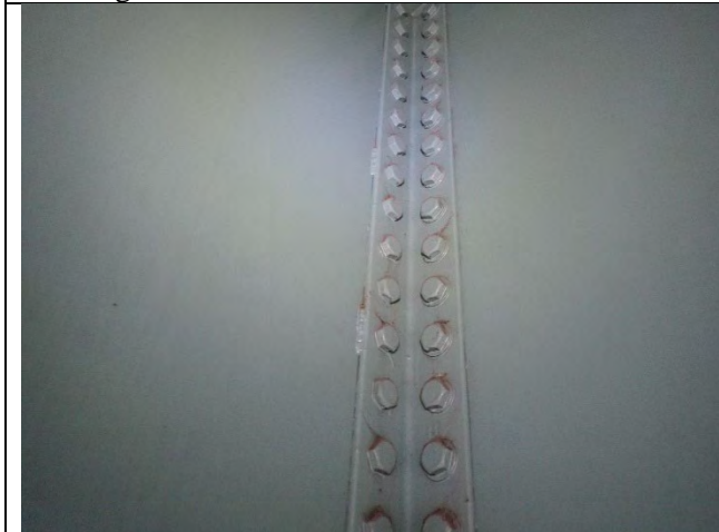
Photograph 28: View of the Typical Tack/Stitch Welds Along the Girder Clip Angle Connection, Looking Southeast.
