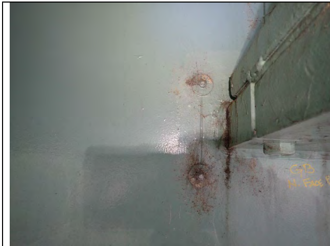
Photograph 26: View of the Typical Drilled Hole Retrofit, North Web Face at Girder B Shown, Looking South.
