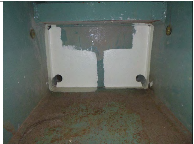
Photograph 25: Typical View of the Coped and Painted Drilled Hole Retrofits at Lower Corners of Diaphragms and Bottom Flange Plate.
