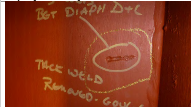
Photograph 8: Typical Gouge in the South Web Between Diaphragms D and E, Looking South.
