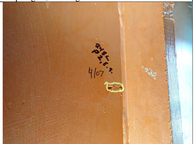
Photograph 19: Gouge at the North Web West of the East Bearing Stiffener, Looking North.
