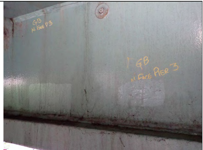
Photograph 27: View of the Ground Off and Painted Tack Weld at the North Web Plate Under Girder B, Looking South.
