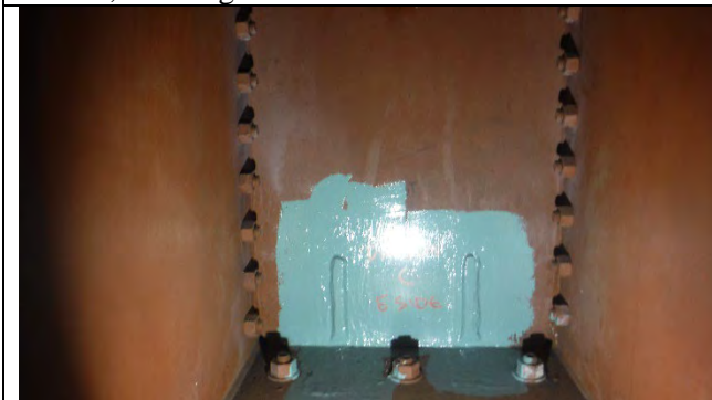
Photograph 6: View of the West Face at Diaphragm A. Typical Example of Removed Knee Braces on Diaphragms, Looking West.
