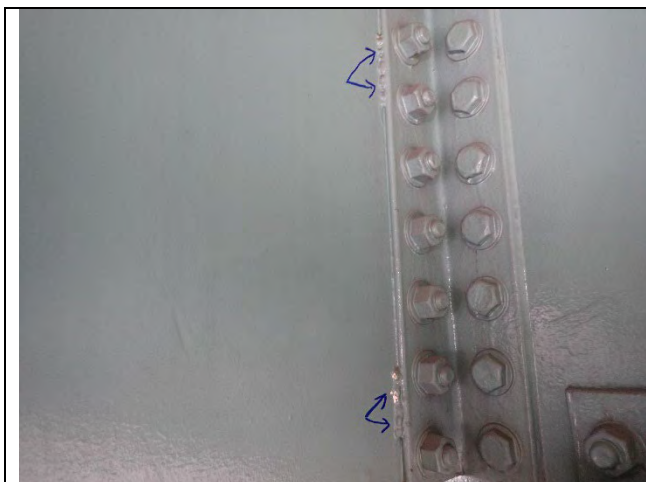
Photograph 20: View of Typical Stitch Welds on Girder to Cap Web Clip Angles., Looking South.
