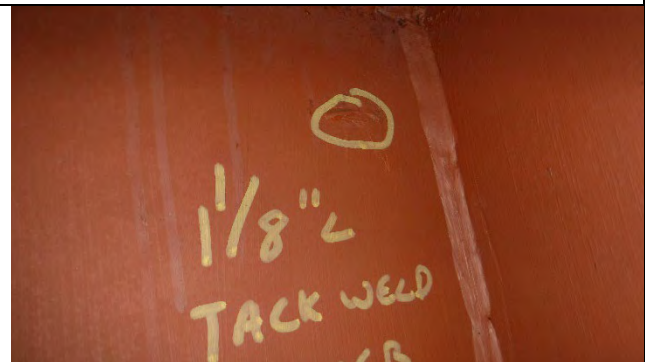
Photograph 7: View of Tack Weld in the North Web Between Diaphragms C and D.
