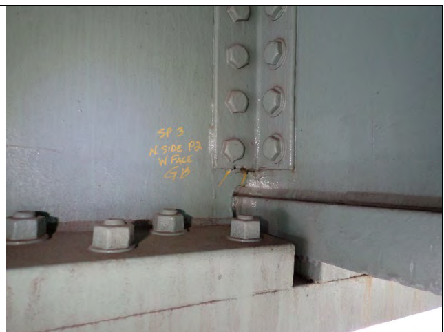
Photograph 21: Two Tack Welds Present Along the Base of the Clip Angle Between the Clip Angle and Girder, Looking West.
