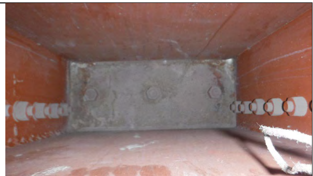
Photograph 5: Typical Steel Pitting at End of Cap, East End Shown.
