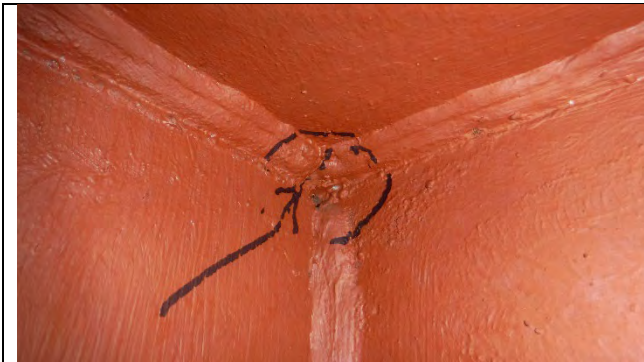
Photograph 10: Weld Porosity Between the Top Flange and the North Web West of Girder F.
