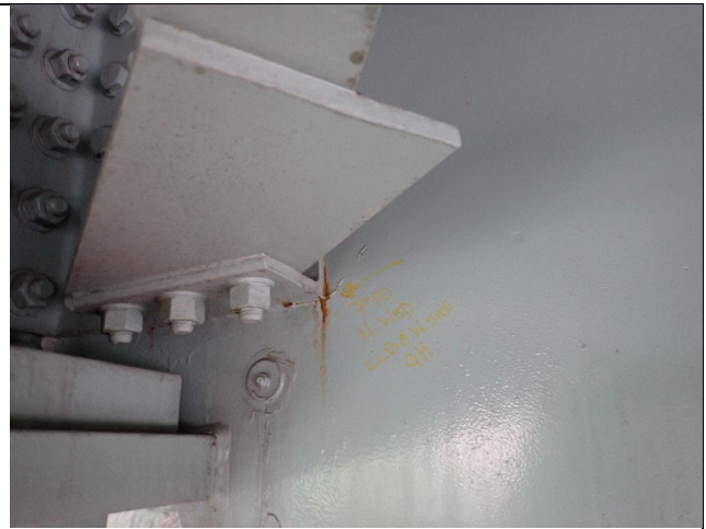
Photograph 29 – View of Minor Fretting Corrosion Between the Bolted Connection on the North Web and Lower lateral Bracing on the East Side Girder G.
