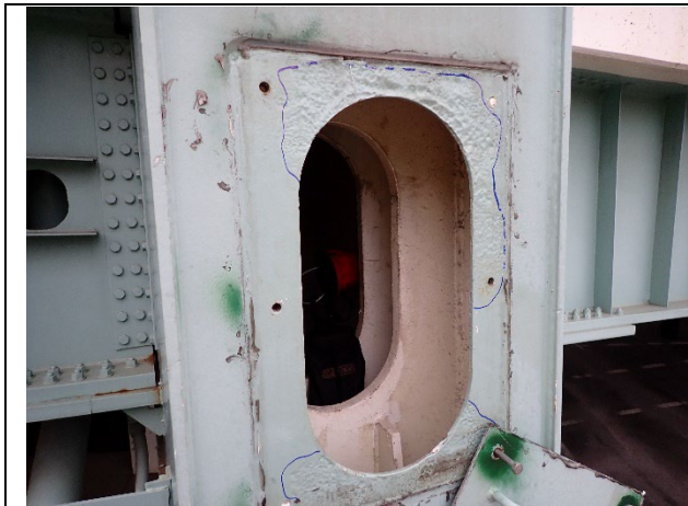
Photograph 22 – View of Painted over Pitting on West End Plate, looking East.
