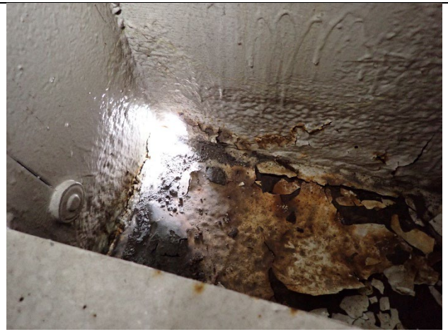
Photograph 6 – View of Laminating Corrosion On The Bottom Plate at the West Hatch
