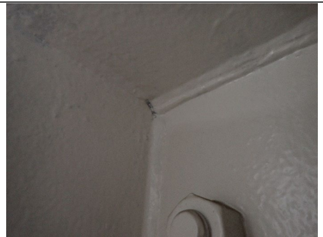
Photograph 23 – View of Top West Corner of Diaphragm D, South Cap Plate. Note Typical Triaxial Weld
