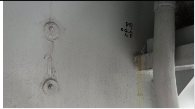
Photograph 31 – View of the Drilled Holes and Sawcut Retrofits Installed 13 in. away from Bottom Flange Tie Plates. Girder A South Side Shown.
