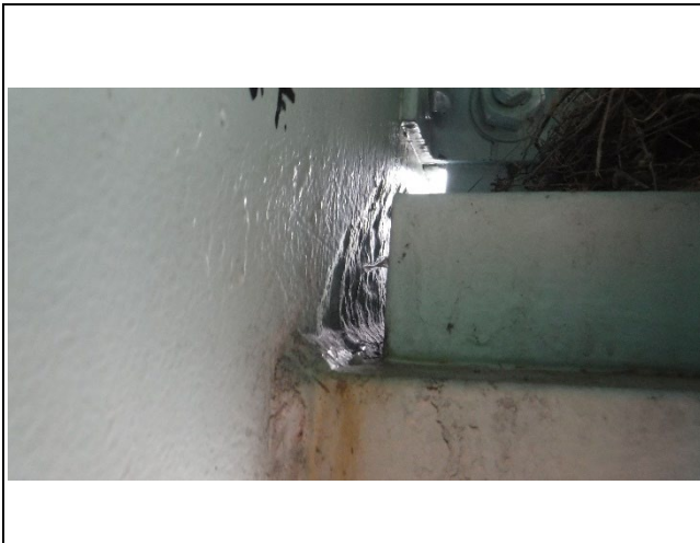
Photograph 28 – View of the Painted over Section Loss on the North Web Plate Behind the Bottom Flange Tie Plate at Girder A. No Change.
