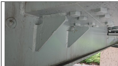
Photograph 51 – General Example of Retrofits to Pier Cap. North Side Girder E Shown.
