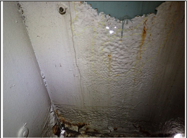
Photograph 4 – View of 3 Corrosion Holes Present at the West end of the Cap Plate.
