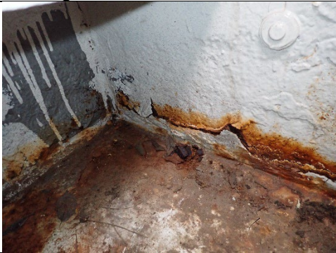
Photograph 45 – View of Reactivating Corrosion and Section Loss on Bottom Cap Plate at West End.
