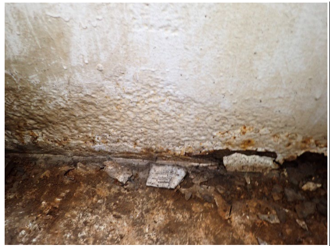
Photograph 10 – View of Painted over Pitting Up To 1/16 in. Deep with Reactivating Laminating Corrosion between the east hatch and Girder J diaphragm.
