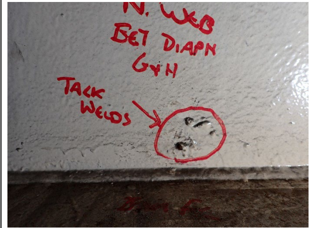
Photograph 27 – View of Typical Tack Weld Present Inside Cap. Base of North Cap Plate Between Girders G and H Shown.
