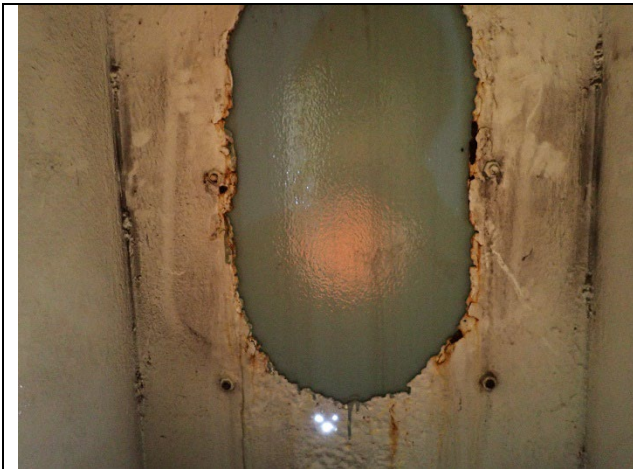
Photograph 5 – View of Knife Edging And Reactivating Laminating Corrosion Around West Hatch
