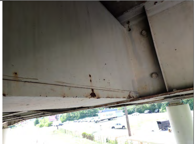
Photograph 13 – General Example of Flaking Paint and Surface Corrosion Along the Pier 3 Cap Edge. Looking Northeast.
