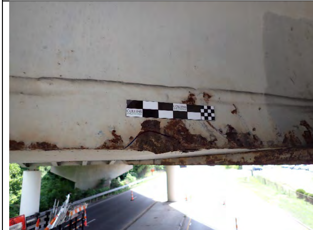
Photograph 18 – Close Up View of 4 in. Long Impact Damage To Cap Bottom Plate, West of Girder 3. Looking Southwest.
