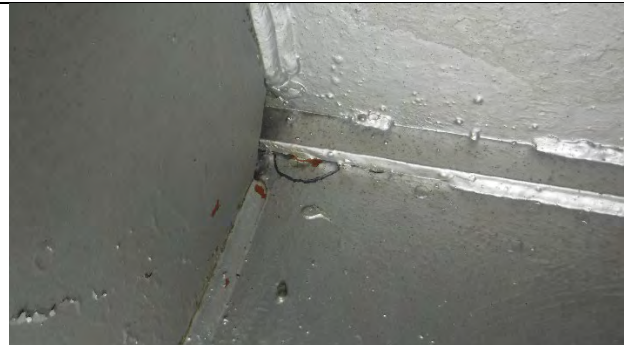
Photograph 5: View of Cracked Tack Weld Between the Top Flange and South Web at Girder 7. Looking South.
