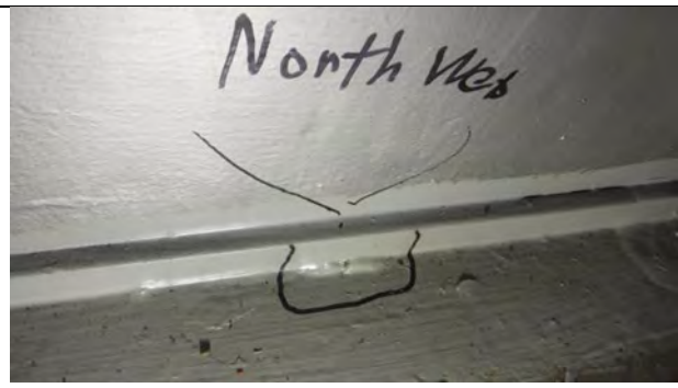
Photograph 7: View of Tack Weld on Cap Bottom Flange at the Cap North Web, East of Girder 3. Looking North.
