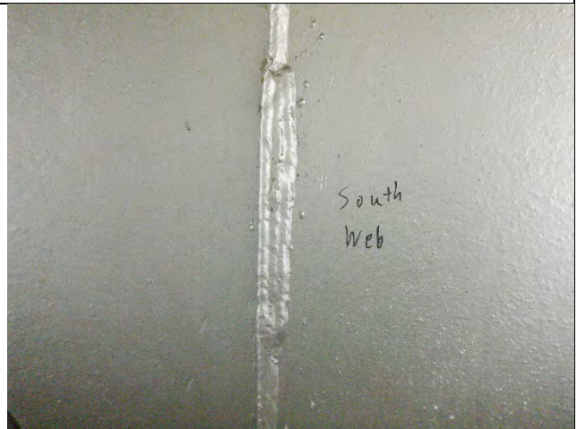
Photograph 23 – General Example of Overlapping Weld for Cap Web Plate to Diaphragm Weld. Looking South.
