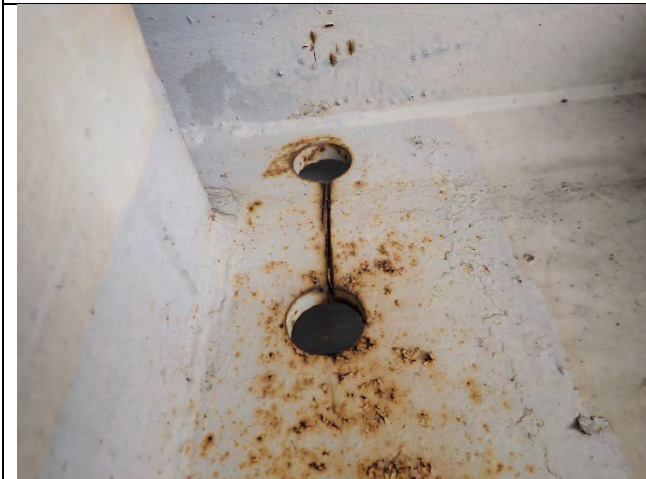
Photograph 14 – View of Two Stress Relief Holes With Errant Sawcuts at the West Face of Girder 2, South Side of Pier. Looking Northeast.
