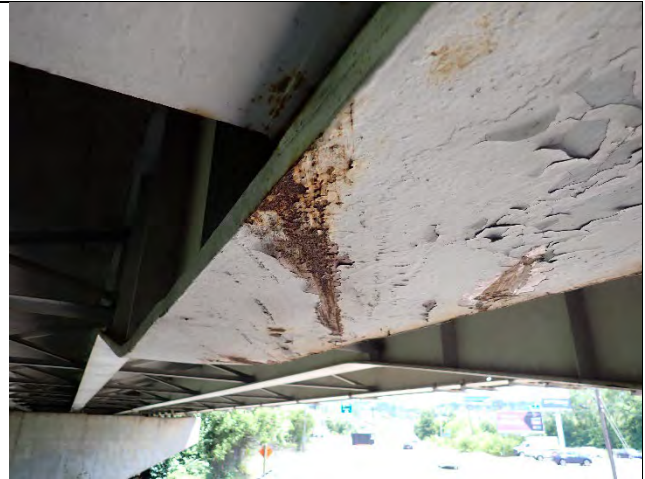
Photograph 27– View of Impact Scrapes and Surface Corrosion On the Underside of the Cap East of Girder 5. Looking Southwest.
