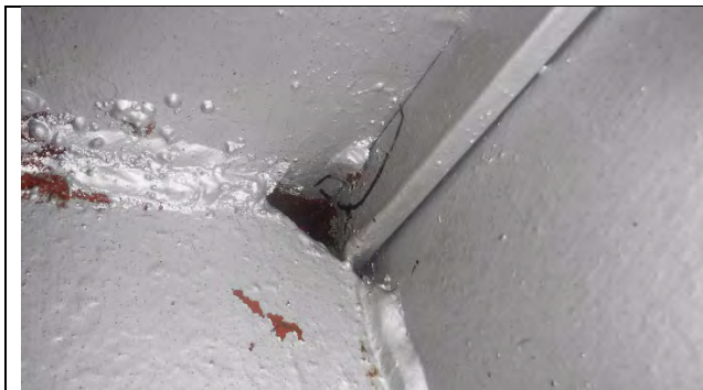
Photograph 6: View of Cracked Tack Weld Between the Top Flange and North Web Between the East Bearing and Girder 7.
