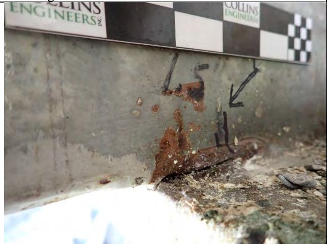
Photograph 15 – Close Up View of a 1-9/16 in. Crack on East Side of Girder 5, North Face of Cap. Note 1/16 in. of Growth. Looking South.
