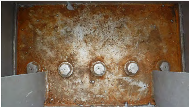
Photograph 4: General Example of Surface Corrosion on the Bottom Flange Adjacent to West Access Hatch. Facing West.
