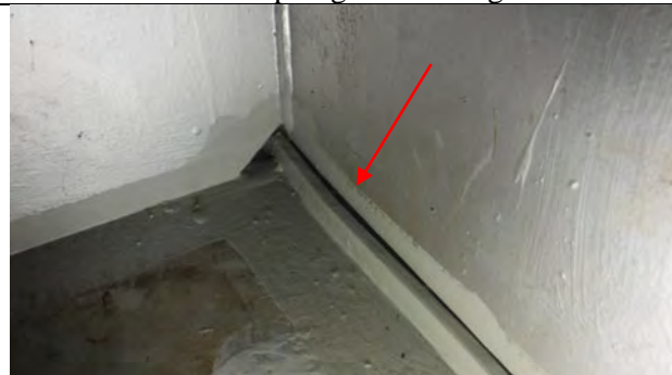
Photograph 11: General Example of Gap Between the Backer Bar and the South Web Plate Located West of the Girder 6 Diaphragm. Looking East.
