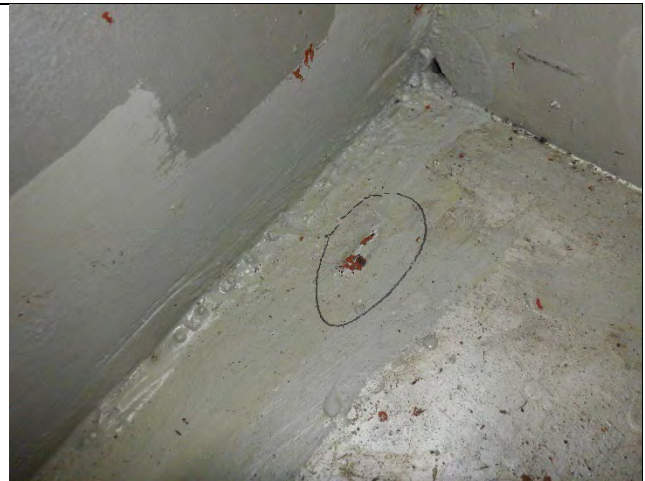
Photograph 25 – View of Partially Ground Down Tack Weld on Cap Bottom Flange West of Girder 5 Diaphragm. Looking East.
