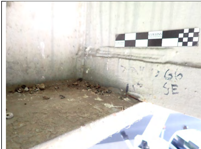
Photograph 16 – Close Up View of a 1-1/2 in. Crack on East Side of Girder 6, South Cap Face. Looking North.
