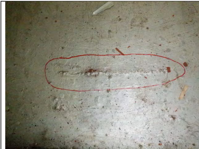
Photograph 24 –View of 7 in. Long Weld on Cap Bottom Flange East of Girder 6 Diaphragm. Looking East.
