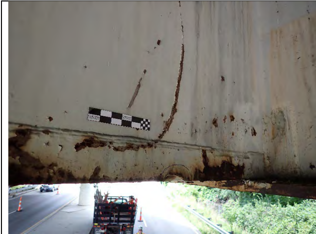
Photograph 26 – View of Impact Gouges and Surface Corrosion On the North Face of the Cap East of Girder 5. Looking Southwest.
