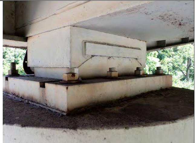
Photograph 19 – View of Typical Bearing Corrosion and Configuration. West Bearing Shown. Looking Northwest.
