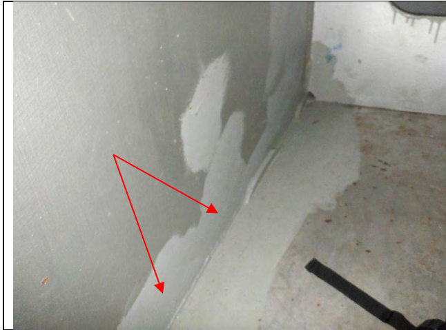
Photograph 20 – General Example of Backer Bar Removed From Cap Bottom Plate. Occurs Along Portions of Cap Interior. Looking Southwest.
