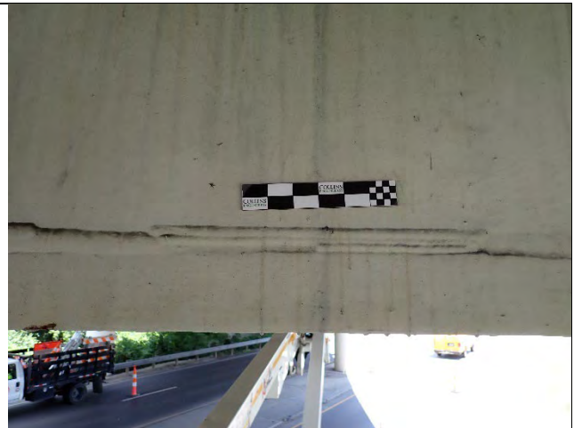
Photograph 17 – General Example of Discontinuous Fillet Welds Not Ground Smooth. Looking North.
