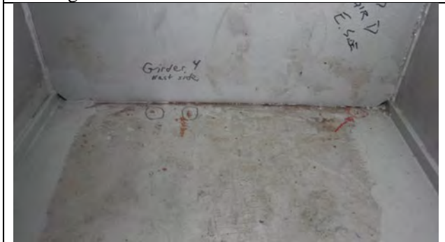
Photograph 8: View of 1/2 in. Tack Welds on the Cap Bottom Flange East Face of Girder 4 Diaphragm. Looking West.
