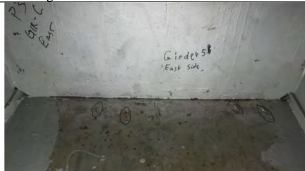
Photograph 9: View of Four Tack Welds Ranging From 1/2 in. to 1 in. on the Cap Bottom Flange East Face of Girder 5 Diaphragm. Looking West.
