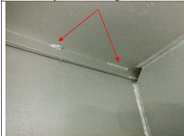
Photograph 22 – Typical Example of Stitch Welds With Varying Lengths Along Cap Top Flange Backer Bars. Looking North.
