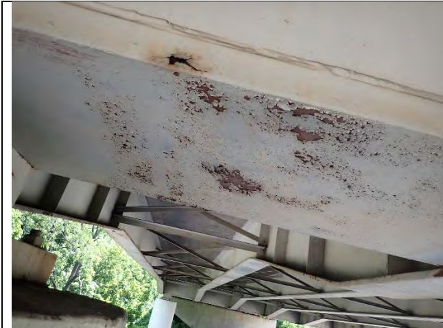
Photograph 12 – General Example of Flaking Paint and Surface Corrosion at Pier 3, Underside Looking Northeast.
