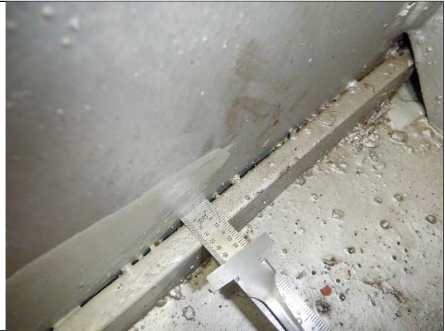
Photograph 21 – General Example of Gap Between Backer Bars and Cap Web Plate. Looking South.
