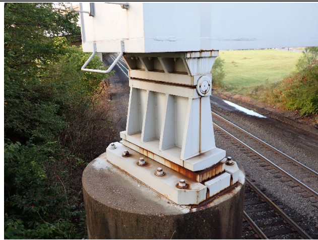
Photograph 22 – View of the Surface Corrosion at the West Bearing.
