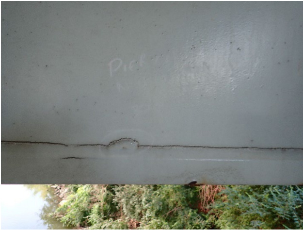
Photograph 8 – View of the Fillet Welds at Groove Weld Between the North Web and the Bottom Flange Weld Between Girder 2 and 3.
