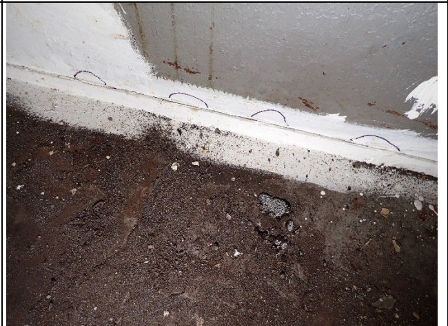
Photo 16 – General Example of the Partially Removed Welds Between the Backer Bar and the Bottom Flange.
