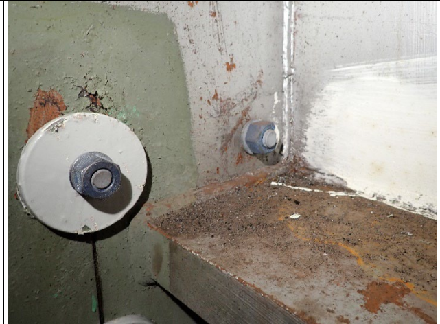
Photograph 20 – General Example of Triaxial (Intersecting) Welds at Cap Web Plates, Tie Plates, and Girder Diaphragms. East Face of Girder 7 at South Web Plate Shown.
