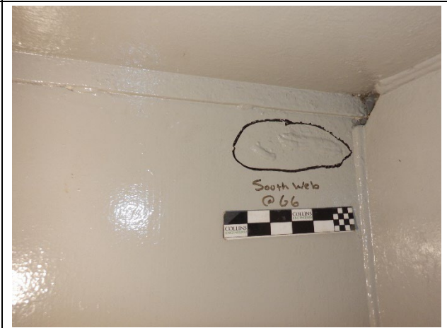
Photograph 7 – Example of a Typical Weld Remnant, East Face of South Web Plate of Girder 6 Shown.
