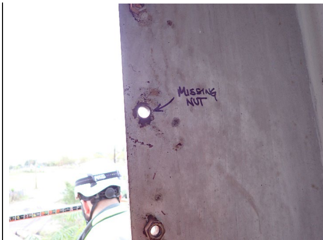
Photograph 13 – View of Missing Hatch Bolt, West Hatch Shown.
