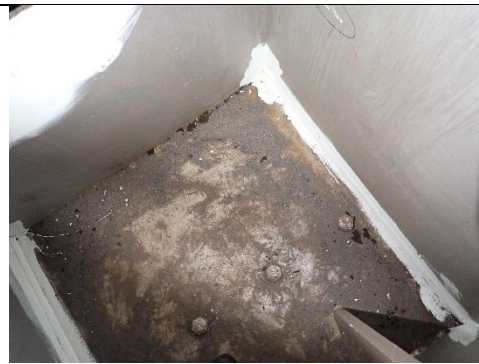
Photograph 28 – View of the Typical Bottom Flange of Pier Cap 20. Note No Major Defects.
