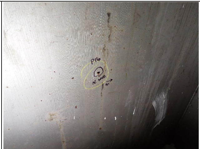
Photograph 18 – View of a Random Tack Weld on the North Web between Girder 1 and the west diaphragm.
