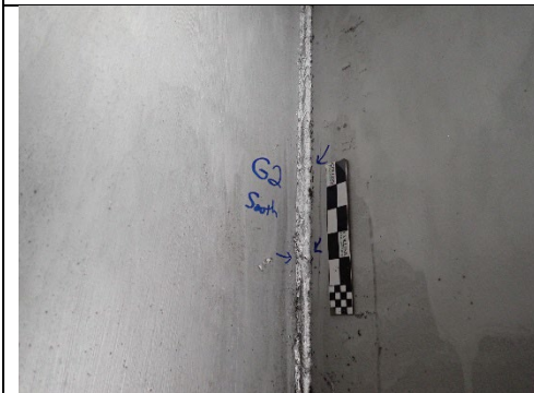
Photograph 33 – General Example of Poor Quality Fillet Welds Between Cap Web Plates and Girder Diaphragms.
