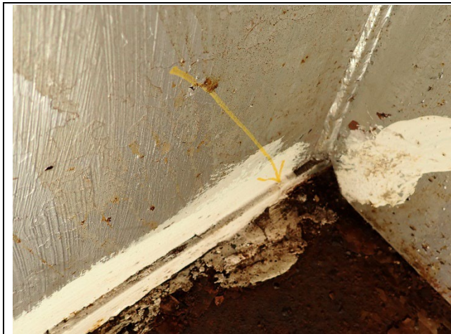
Photograph 17 – View of the Isolated Portions of Backer Bar Removed Along the Length of the Pier Cap to eliminate Butt Joints.
