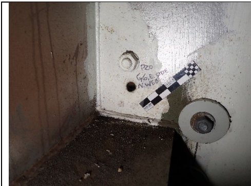
Photograph 31 – View of the Unfilled Stress Relief Hole above the Girder Bottom Flange East of Girder 6 at the North Web.
