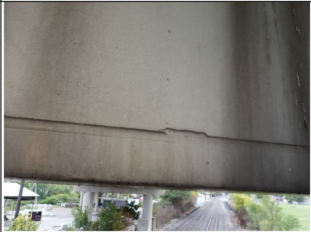
Photograph 25 – General Example of Overlapping Weld Beads within the Full Penetration Welds between the Cap Web Plates and Bottom Flange Plate.
