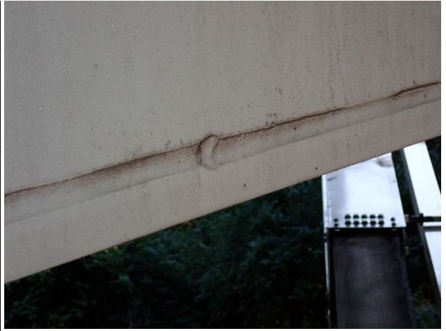
Photograph 9 – View of Typical Overlapping Weld Beads on the Bottom Flange Plate, South Web Below Girder 4 Shown.
