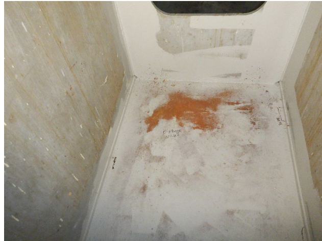
Photograph 4 – View of Typical Surface Corrosion on the Bottom Flange Plate, Between Girders 3 and 4 Shown.
