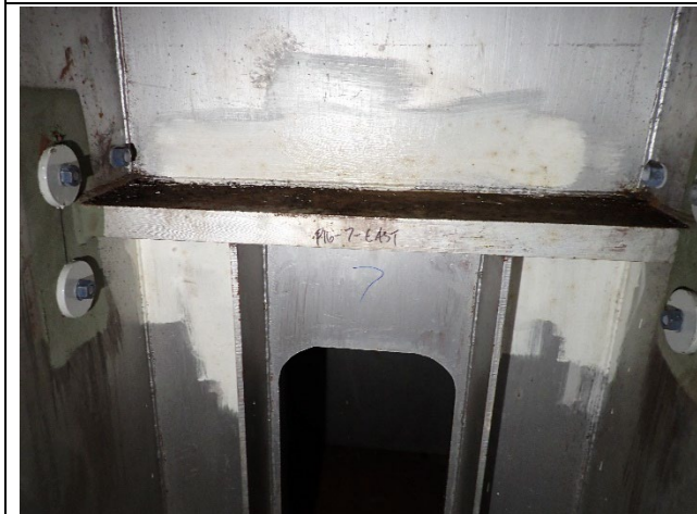
Photograph 21 – View of the Drilled and Bolted Stress Relief Holes Installed in the Pier Cap Web Plates Adjacent to Girder Diaphragms near the Girder Tie Plates.
