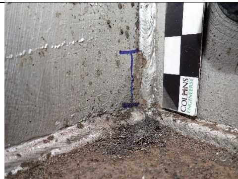
Photograph 34 – View of the 1-5.8 in. Triaxial Weld Crack at the West Face of the Girder 1 Diaphragm at the South Web Plate. Close up view.
