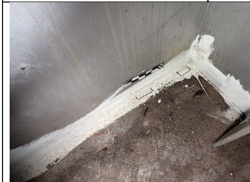
Photograph 29 – General Example of Partially Ground Fillet Welds on Bottom Flange Backer Bar Retrofit.
