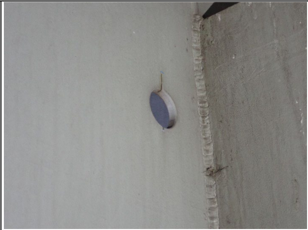
Photograph 23 – View of Typical Drilled Stress Relief Hole with Saw Cuts, North Face of West Side of Girder 4 Shown.
