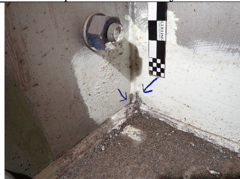
Photograph 30 – General Example of Triaxial Welds at the Intersections of Cap Web Plates, Girder Diaphragms, and Bottom Flange Tie Plates.
