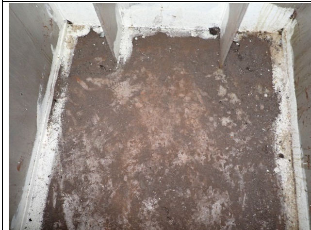
Photograph 15 – View of Accumulation of Steel Filings, Paint Flakes, and Sand Blasting Medium on the Floor.
