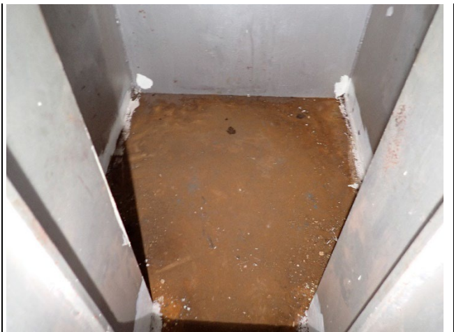
Photograph 14 – View of the Typical Missing Paint and Surface Corrosion, Inside Cap Between Girders 1 and 2 Shown.
