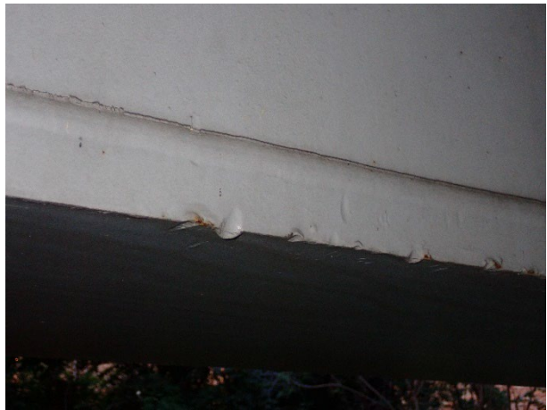
Photograph 10 – View of the Gouges from Construction on the North Face of the Bottom Flange at Girder 2.
