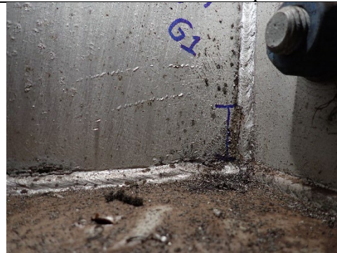
Photograph 36 – View of the 1-5.8 in. Triaxial Weld Crack at the West Face of the Girder 1 Diaphragm at the South Web Plate. Close up view.
