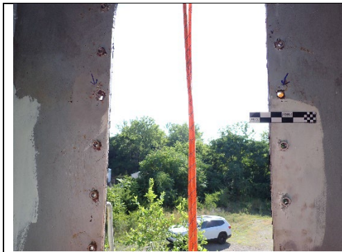
Photograph 27 – Typical Example of Missing Nuts at the East Access Hatch of Pier Cap 20.
