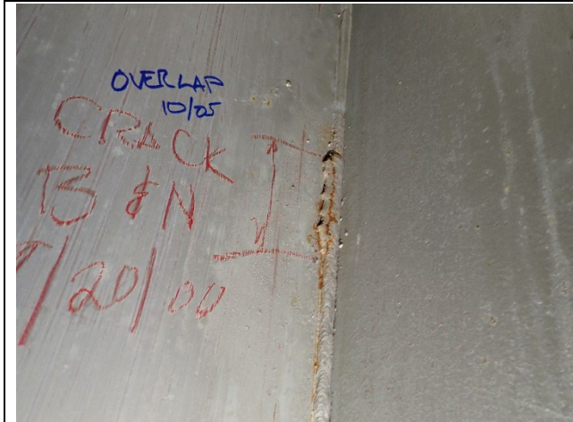
Photograph 19 – View of Excessive Weld Material Breaking off of Cap Web Stiffener, West Side of Diaphragm B Shown.
