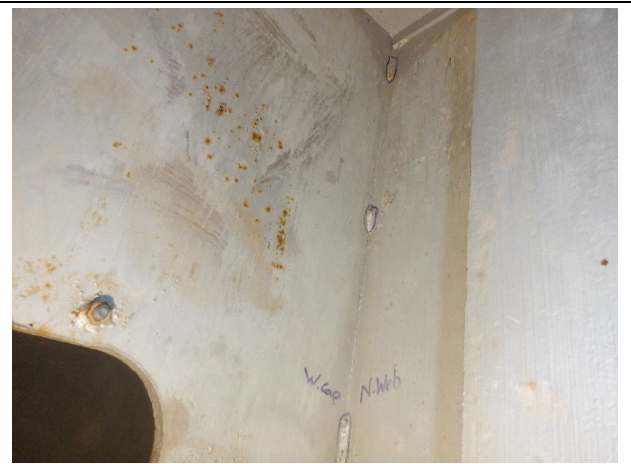
Photograph 6 – View of the Tack Welds Between the North Web Plate and West End Cap.
