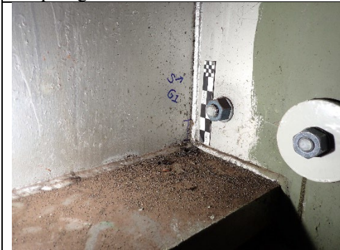
Photograph 35 – View of the 1-5.8 in. Triaxial Weld Crack at the West Face of the Girder 1 Diaphragm at the South Web Plate. Perspective view.
