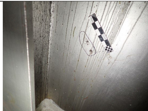
Photograph 32 – General Example of an Unground Tack Weld.
