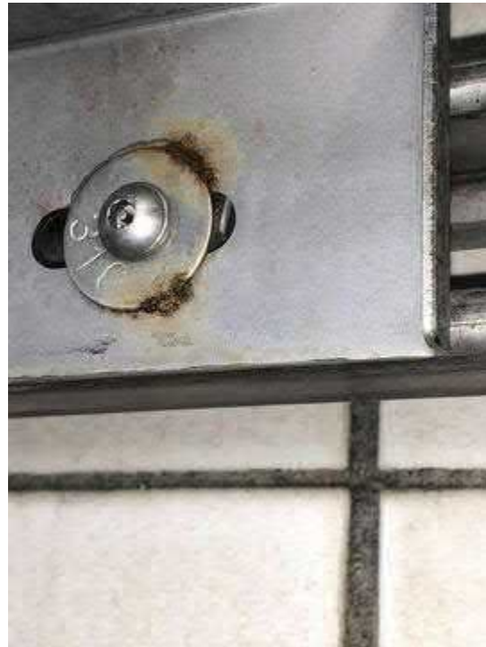
Tunnel Lighting Section
