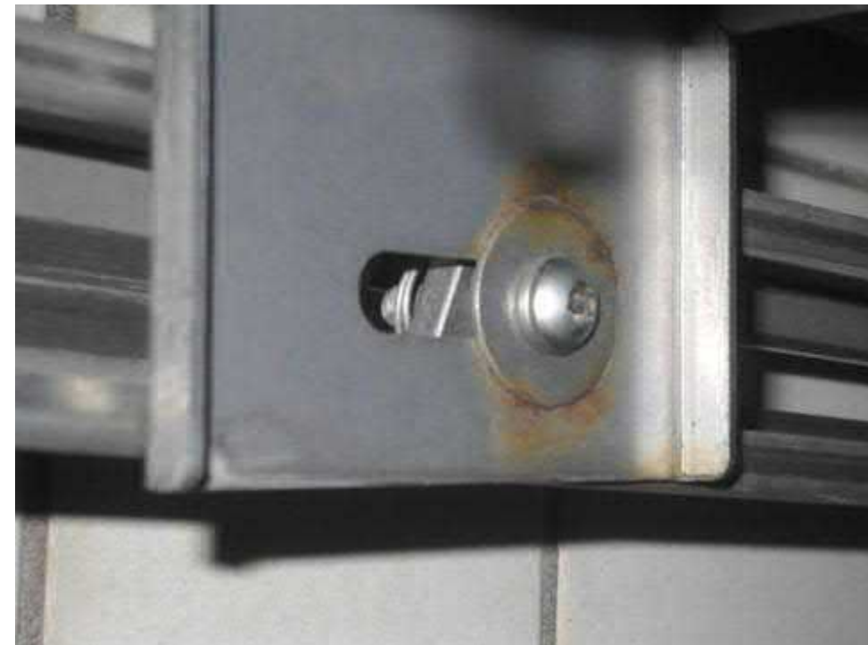
Tunnel Lighting Section
