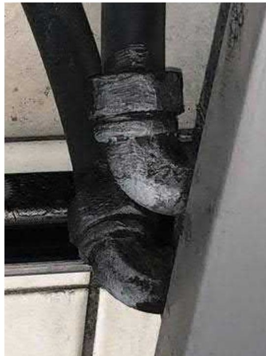
Tunnel Lighting Section
