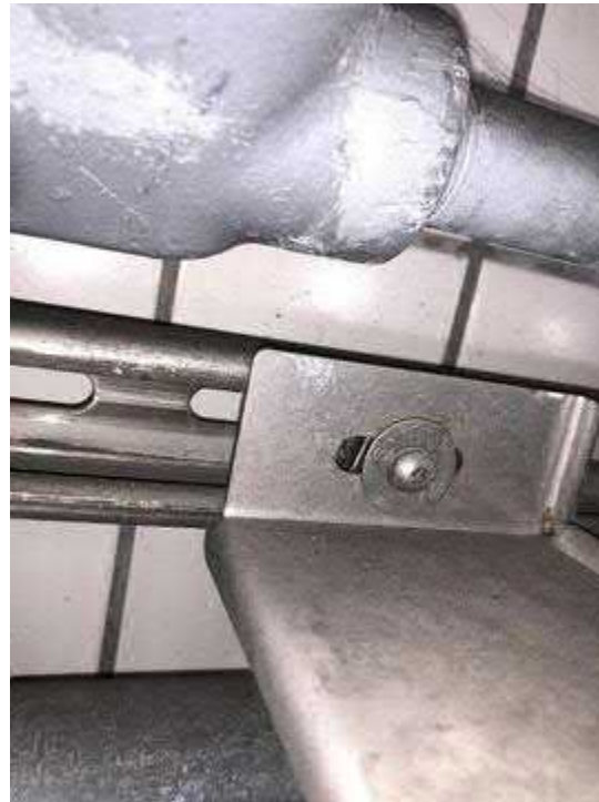
Tunnel Lighting Section
