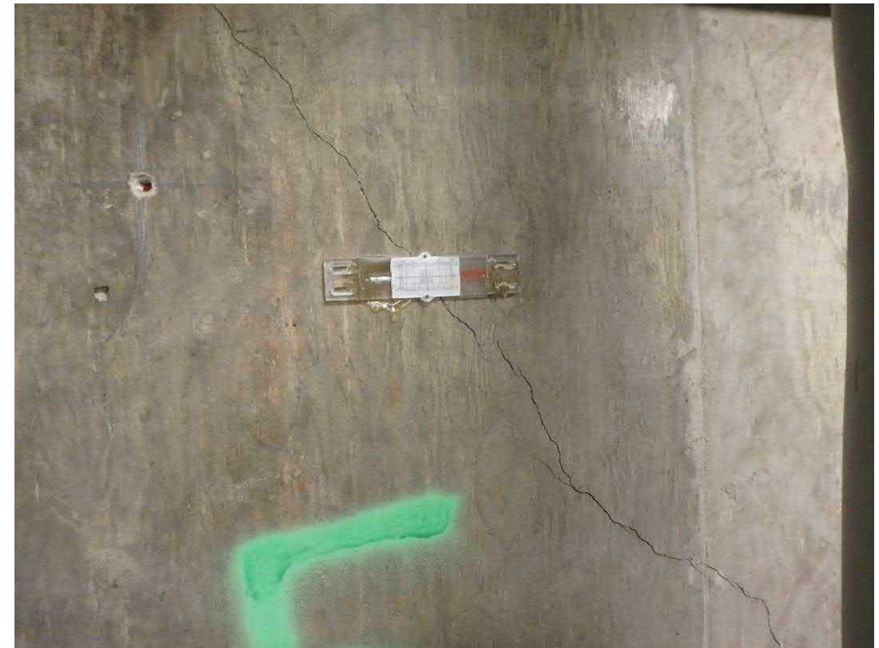
3-8 10 LF Diagonal Hairline Crack with Strain Gauge on Control Room East Wall
