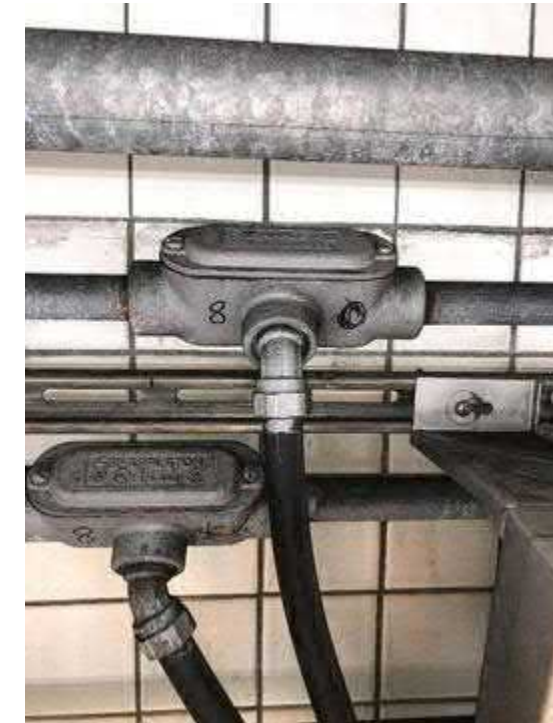
Tunnel Lighting Section
