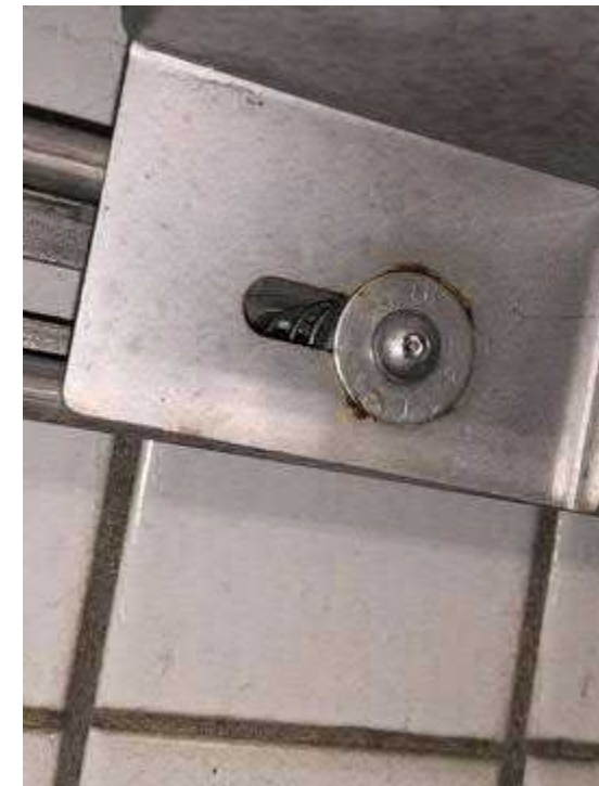
Tunnel Lighting Section
