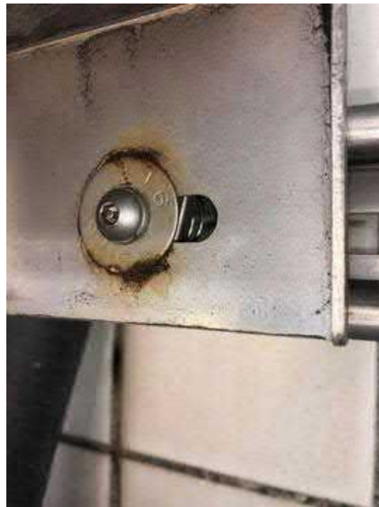
Tunnel Lighting Section
