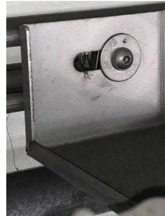
Tunnel Lighting Section
