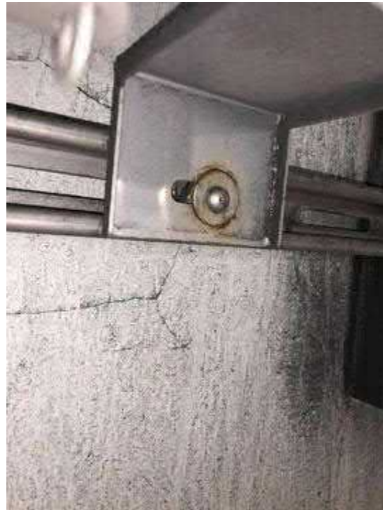
Tunnel Lighting Section
