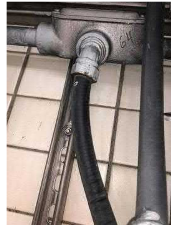
Tunnel Lighting Section
