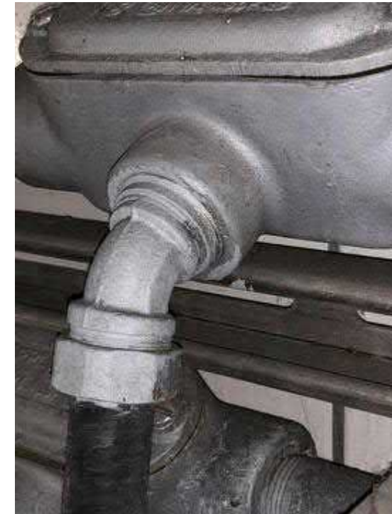
Tunnel Lighting Section
