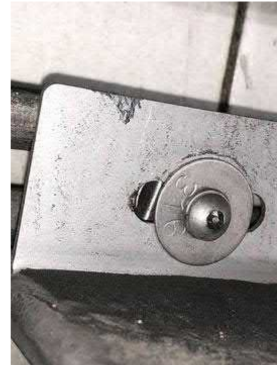
Tunnel Lighting Section
