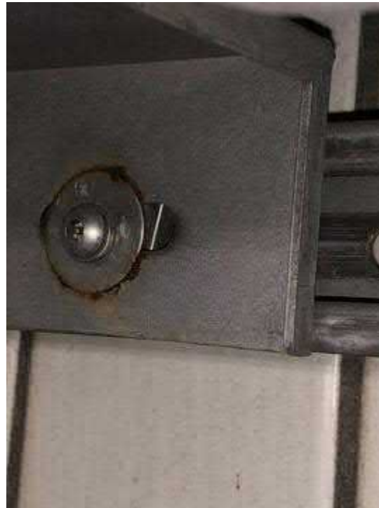
Tunnel Lighting Section
