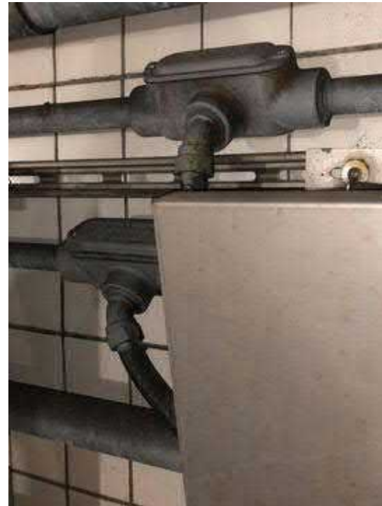
Tunnel Lighting Section
