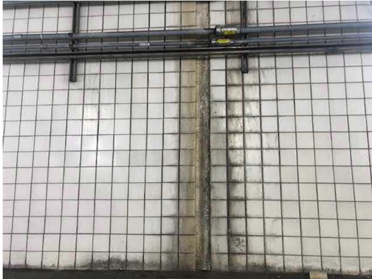
3-9 Large Area of Efflorescence Present Between Units 16/17 in the Ramp Barrel
