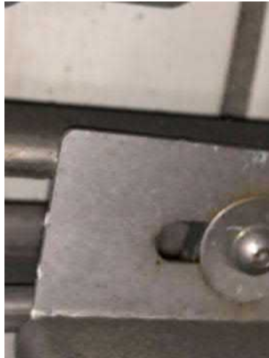
Tunnel Lighting Section
