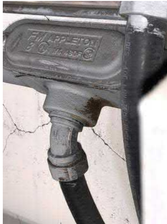
Tunnel Lighting Section
