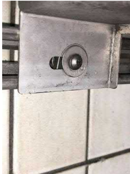
Tunnel Lighting Section
