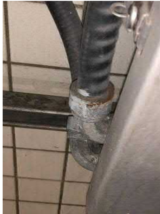
Tunnel Lighting Section
