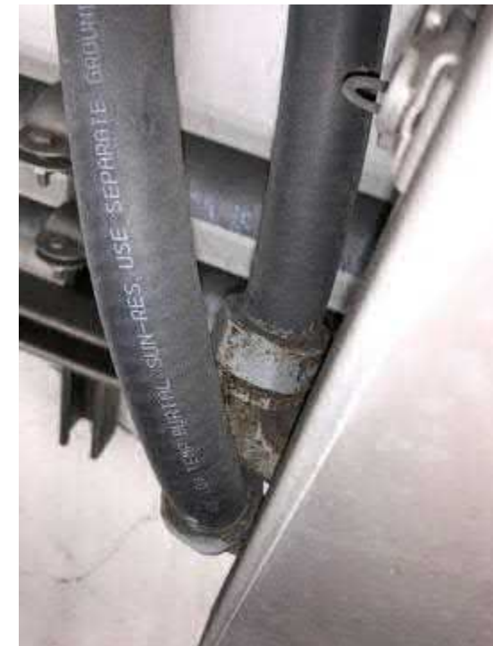
Tunnel Lighting Section
