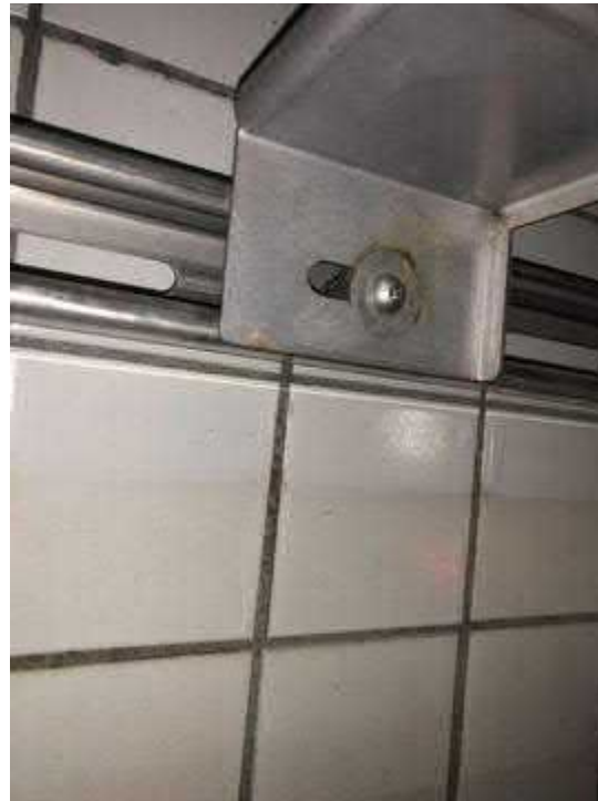
Tunnel Lighting Section
