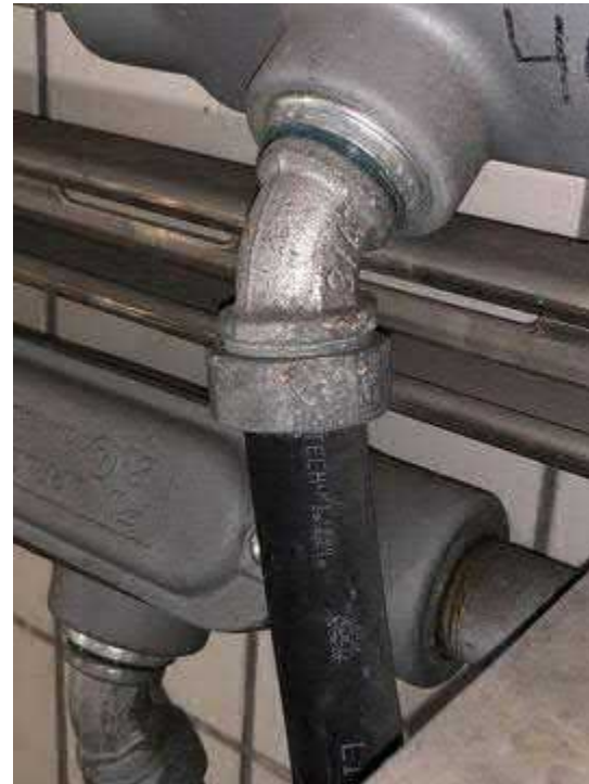
Tunnel Lighting Section
