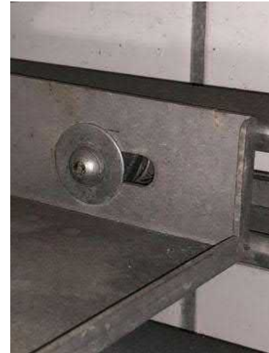
Tunnel Lighting Section
