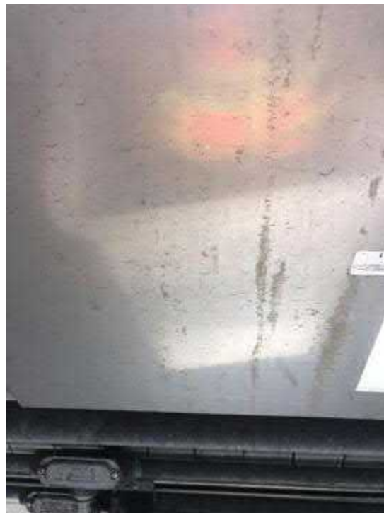
Tunnel Lighting Section
