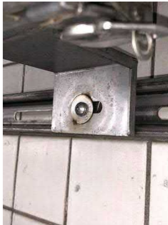
Tunnel Lighting Section
