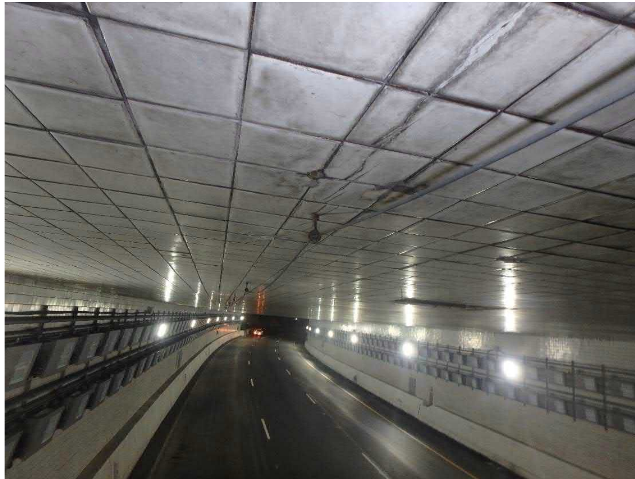
3-7 Typical Hairline Crack in Ceiling Tiles
