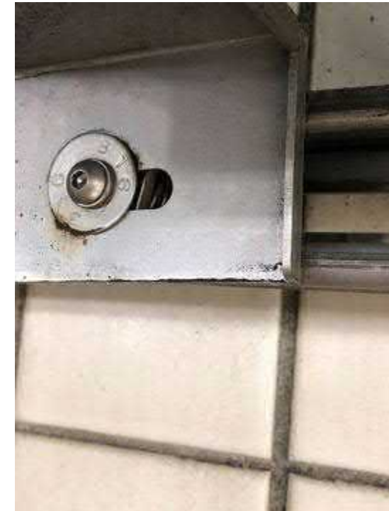
Tunnel Lighting Section
