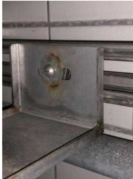
Tunnel Lighting Section
