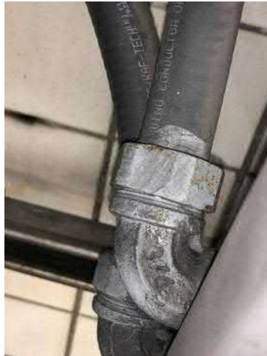
Tunnel Lighting Section
