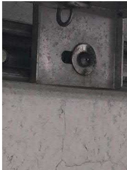
Tunnel Lighting Section
