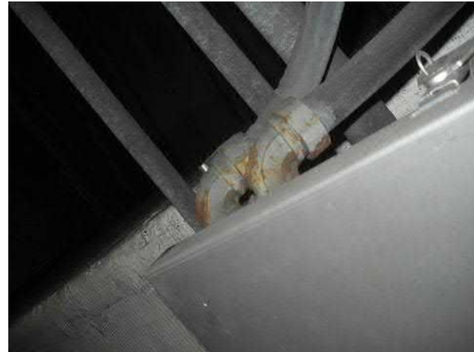
Tunnel Lighting Section
