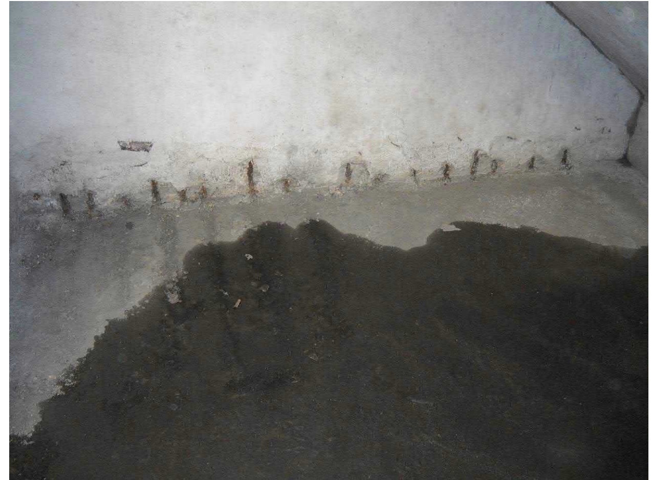
3-10 Area of Delamination and Spalling with Exposed Rebar in Cross Passageway
