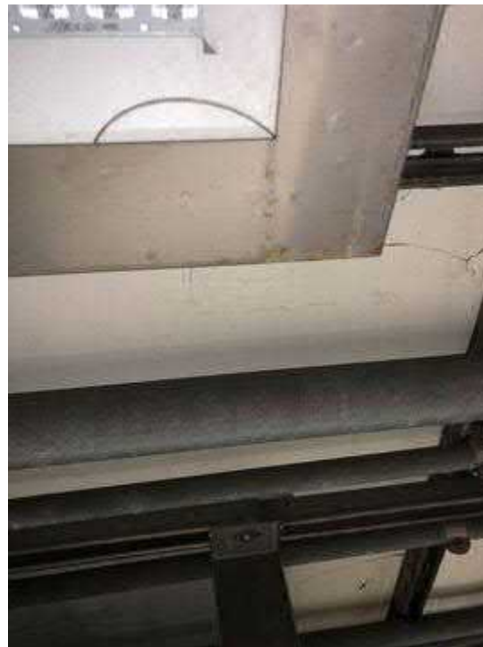
Tunnel Lighting Section
