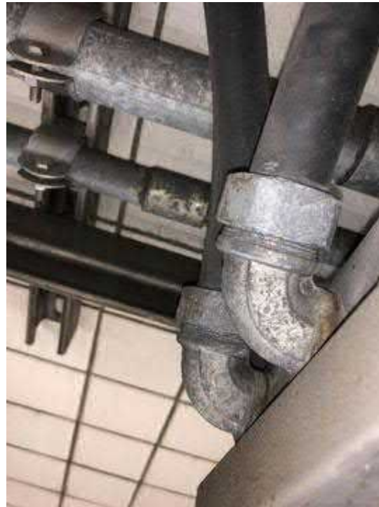
Tunnel Lighting Section
