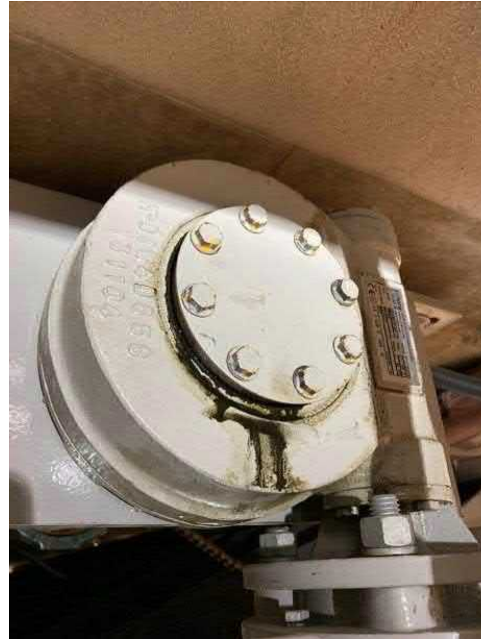
3-1 Damper Actuator Oil Leak
