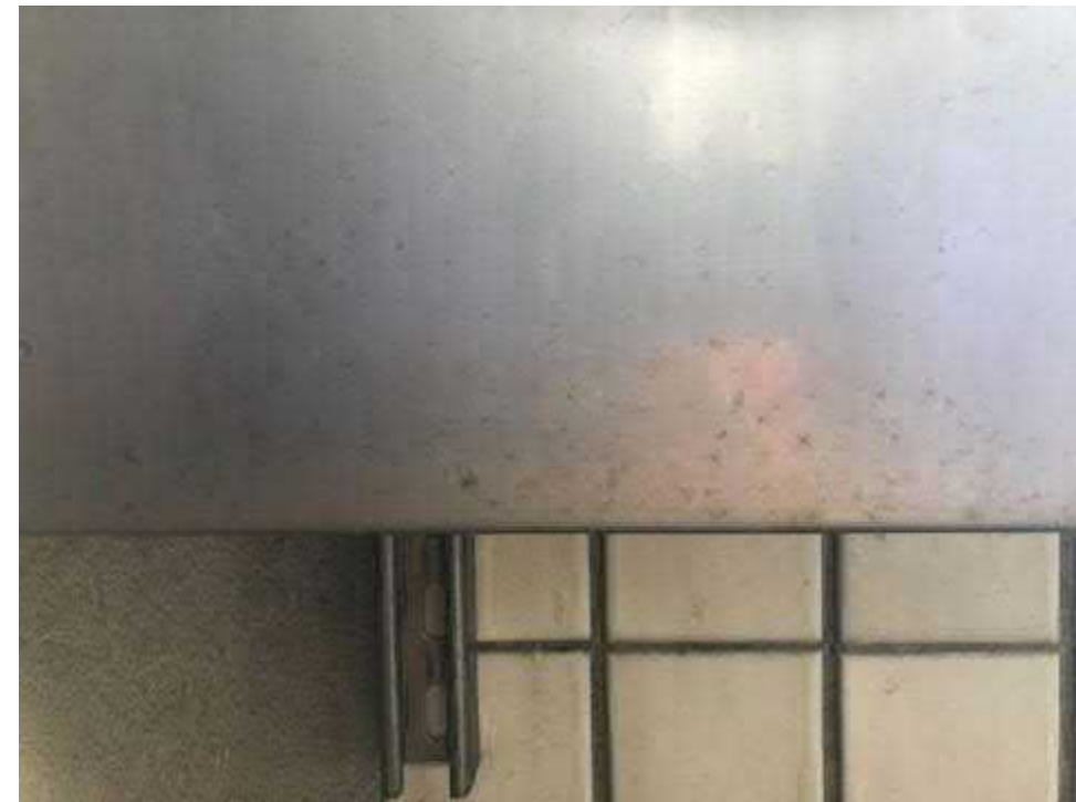
Tunnel Lighting Section
