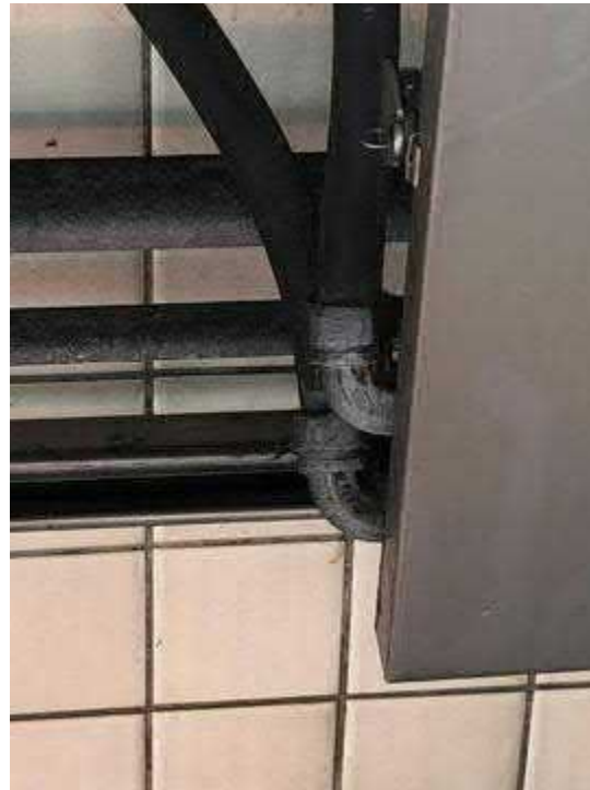
Tunnel Lighting Section
