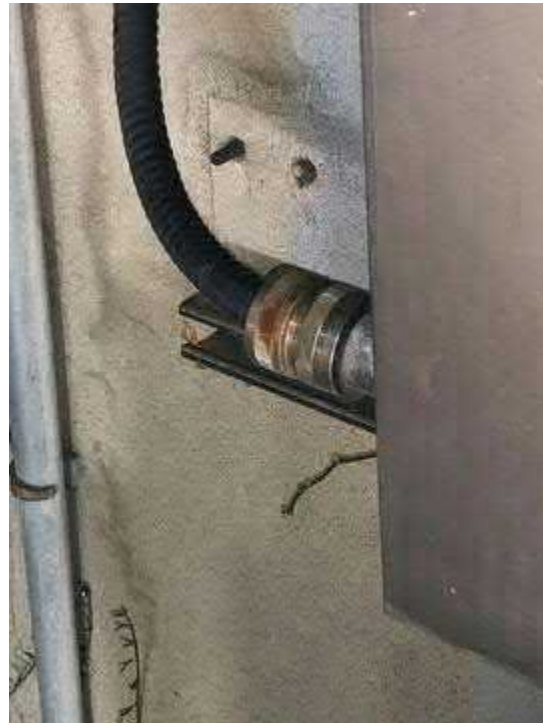
Tunnel Lighting Section
