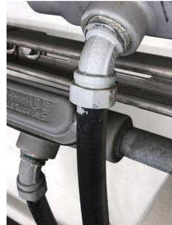
Tunnel Lighting Section
