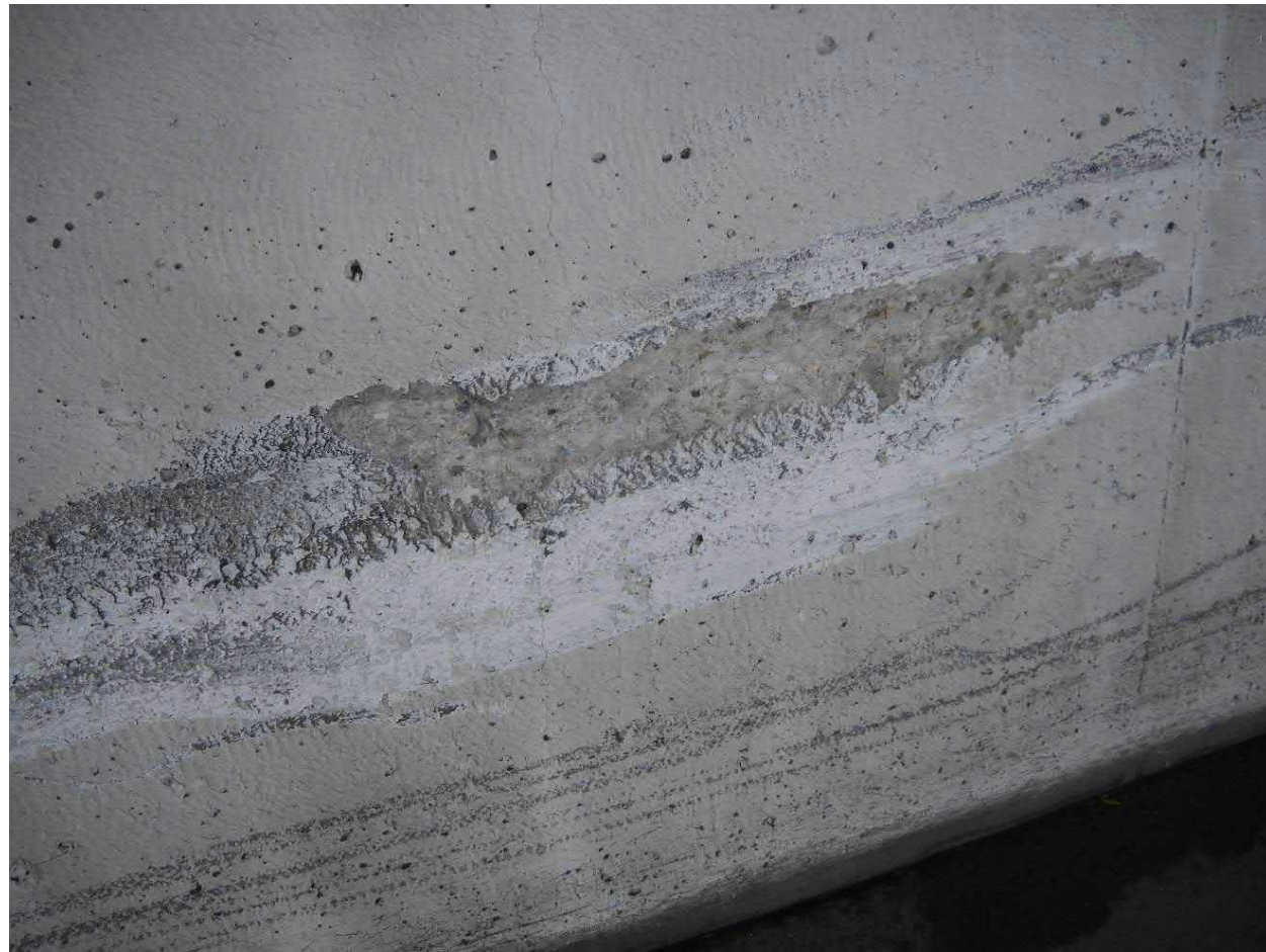
3-12 Typical Vertical Hairline Crack in Barrier and Collision Scrapes
