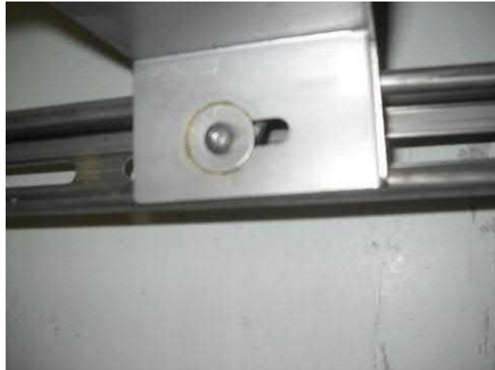
Tunnel Lighting Section
