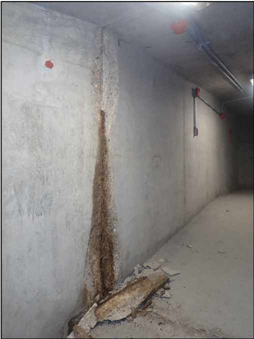
Photo B-1: Spall in north wall at west end of hallway from main access stairs with active leakage, looking northeast
