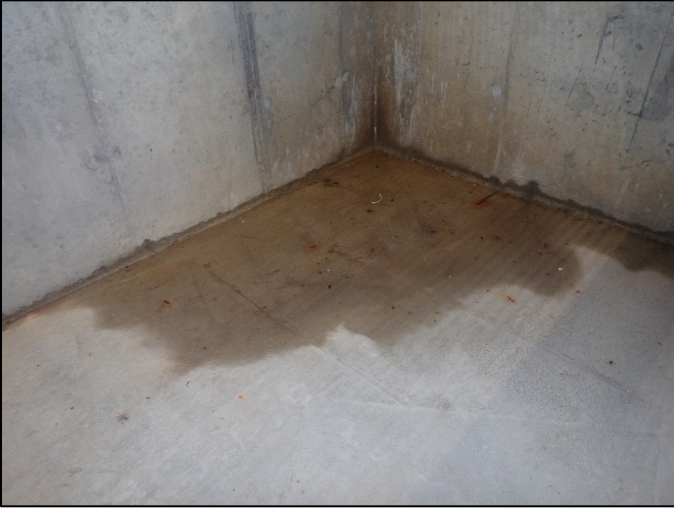
Photo B-5: Standing water in southeast corner of southeast stairway to plenum space, looking southeast
