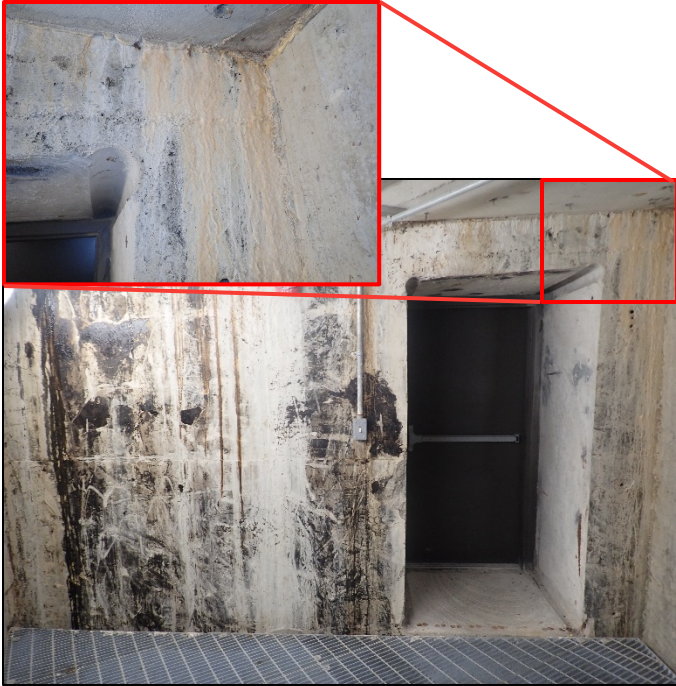
Photo B-4: Heavy efflorescence on top of west wall above door in southeast stairway to plenum space, looking west
