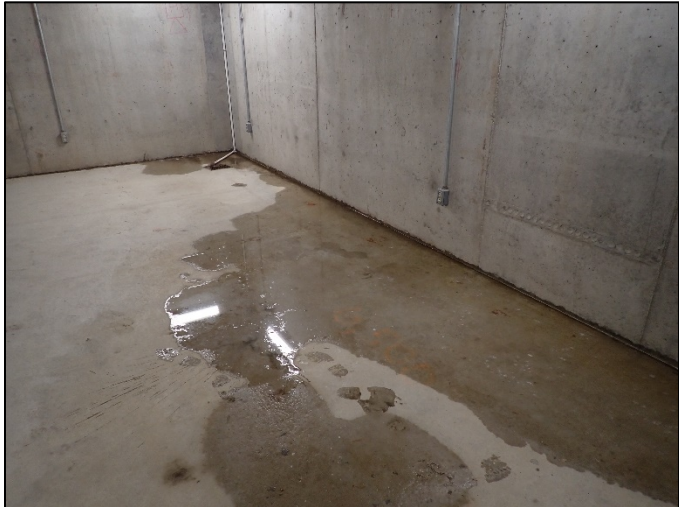
Photo B-7: Standing water along east wall in room between new electrical room and ventilation space, looking northeast
