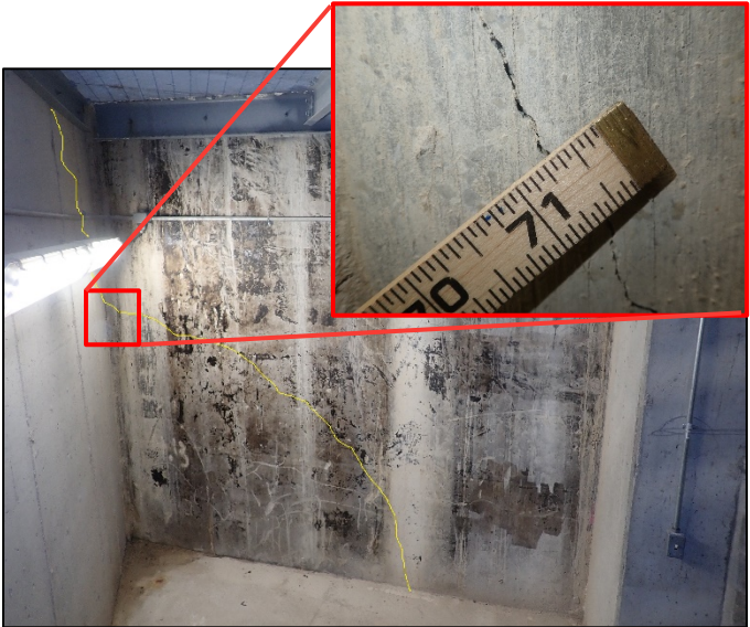
Photo B-6: 1/16" wide crack (highlighted in yellow) in south and west walls of southeast stairway to plenum space, looking west
