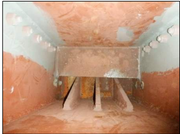
Photo 6: Typical Pitting on Bottom Flange and Bottom of Webs
