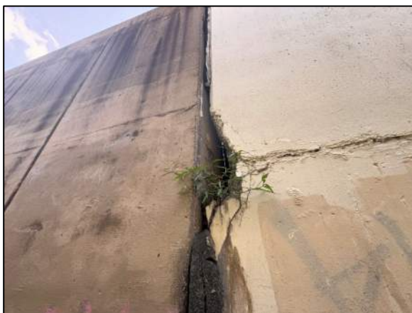
Photo 57: 5' H x 3" L Spall in SE Wingwall Of Abutment 1
