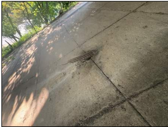
Photo 42: Abutment 2 Slope Protection Drainpipe Section Loss
