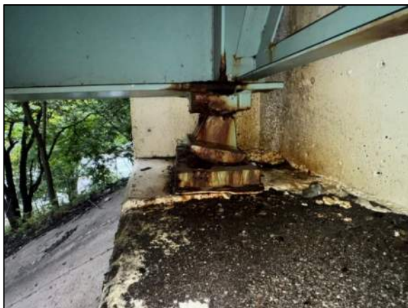
Photo 47: Corrosion and Staining in Rocker Bearing
