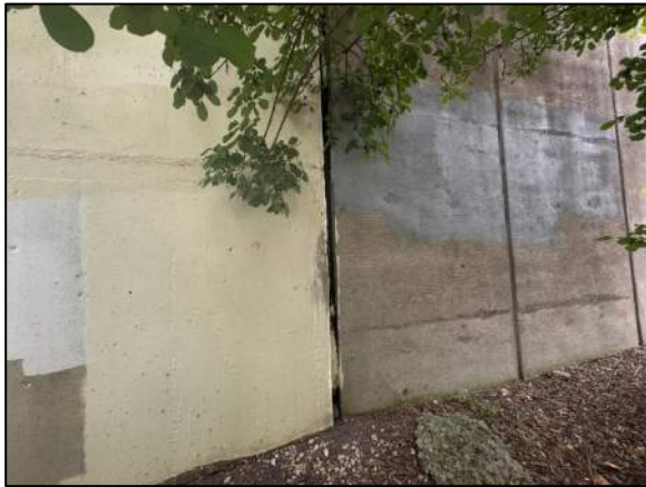
Photo 56: Cracking and Efflorescence in SW Wingwall of Abutment 1
