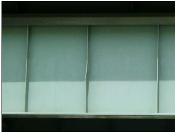
Photo 45: Bent Web Stiffener in Span 3 On Girder G
