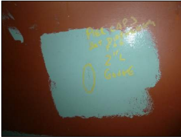
Photo 17: 2" L Gouge Between Diaphragm F and E, North Web
