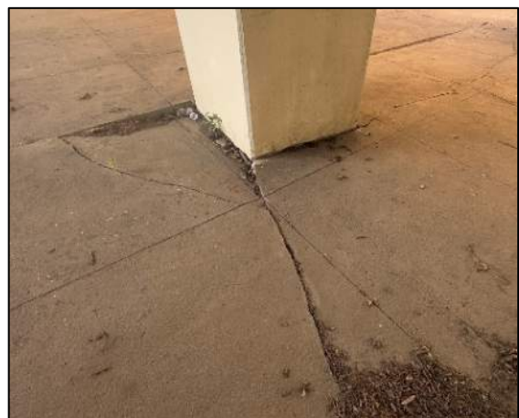
Photo 59: Settlement of slope protection at Pier 1
