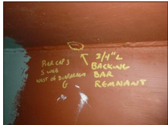
Photo 15: 3/4" Backer Bar Remnant Between South Web, Top Flange, West of Girder G Diaphragm
