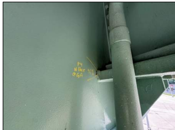
Photo 35: 3/4" H X 1/8" D Inclusion of Fillet Weld Between East Side of Girder A Bottom Flange and North Web
