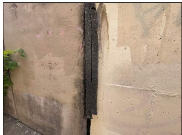
Photo 55: Abutment 1 SE Wingwall Protruding Joint Filler
