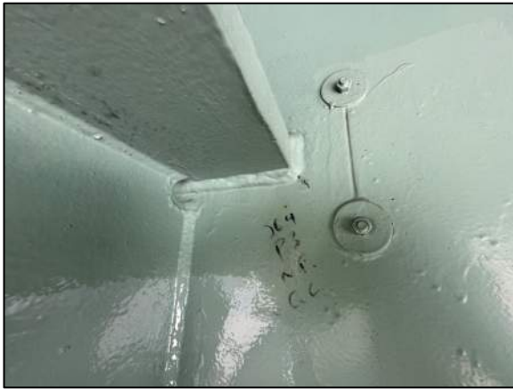
Photo 25: Fillet Weld Porosity at Bottom Flange of Girder C and North Web
