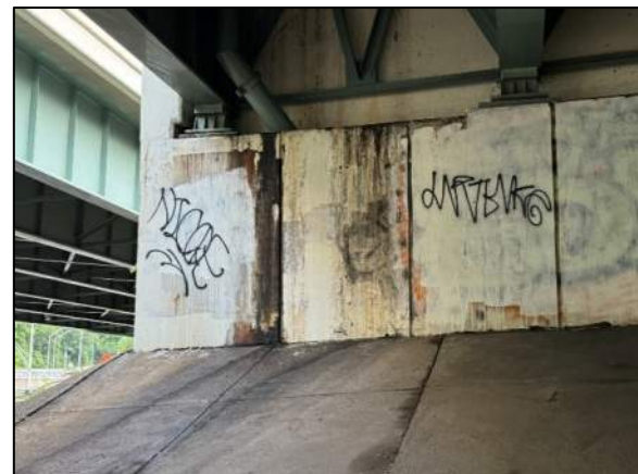
Photo 50: Rust Staining from Drainage Block Along Abutment 1
