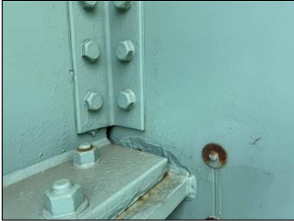
Photo 24: 7" L X 2" H Area of Up To 3/16" Section Loss in South Web and Girder G Tie Plate
