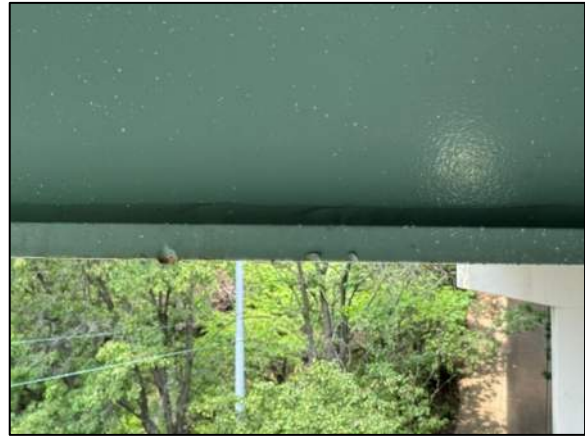
Photo 34: Shallow Gouges Along North Edge of Bottom Flange at Cantilevered Section
