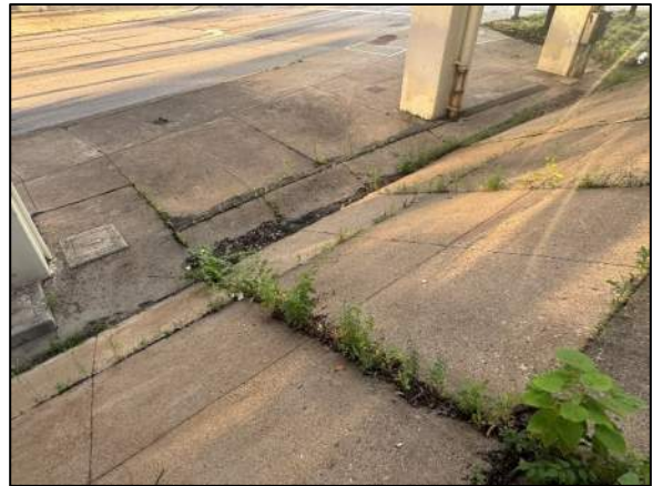
Photo 58: Vegetation Growing Through Joints at Abutment 2 Slope Protection
