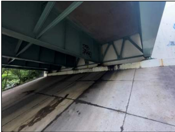
Photo 51: Rust Staining on Stem and Abutment Seat Due to Leaking Deck Joint
