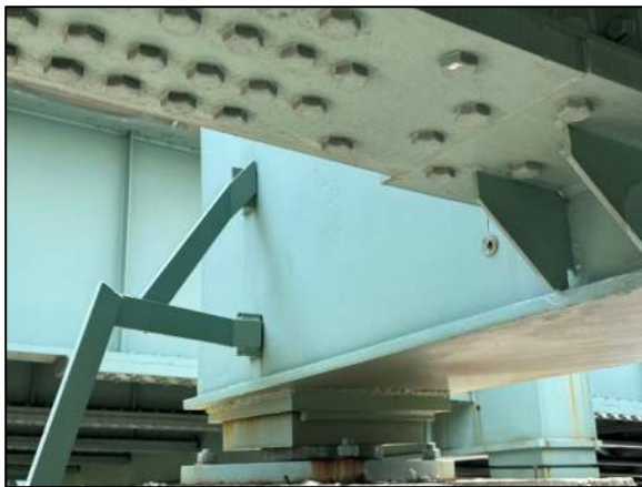
Photo 7: Typical condition of lower flange of steel cap
