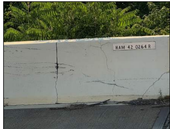
Photo 39: Typical Cracking and Scrapes on Rail
