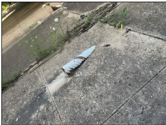
Photo 43: Abutment 2 Slope Protection Drainpipe Section Loss
