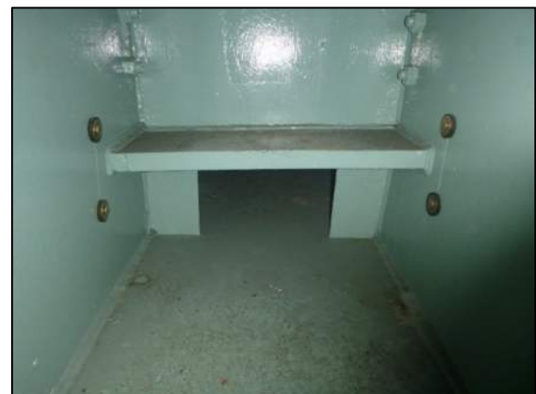
Photo 21: Painted Interior; Bottom Flange and Web. Typical Dog-Bone Retrofit
