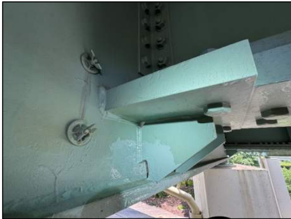
Photo 12: North Web, Knee Brace, retrofit below Girder C. Undercut Welds at Bottom of Knee Brace
