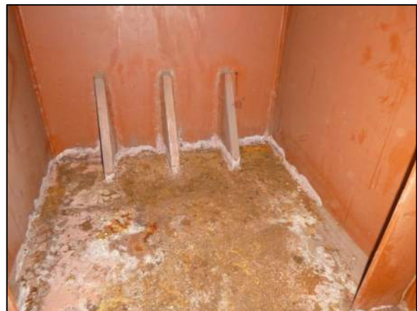
Photo 28: Pooling Water Caused Active Corrosion at West End Bottom Flange and Lower Webs
