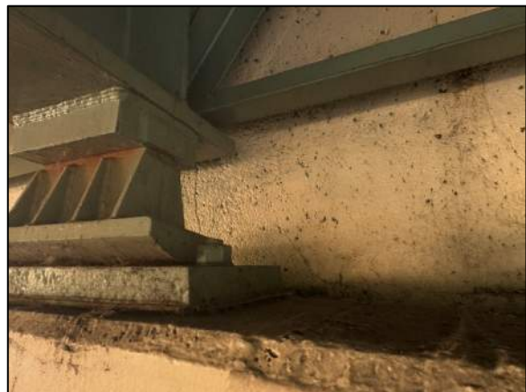
Photo 54: Abutment 2 Back Wall Vertical Cracking
