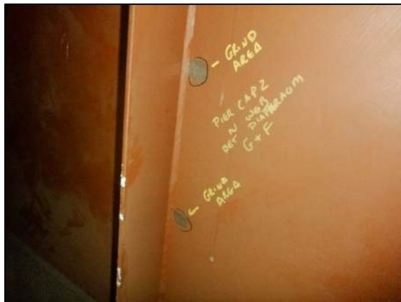
Photo 4: Removed Tack Weld, Ground Area Left Unpainted on North Web Between Girder G and F
