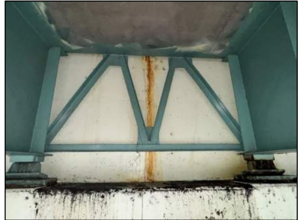
Photo 53: Leakage Staining on Abutment 2 Backwall
