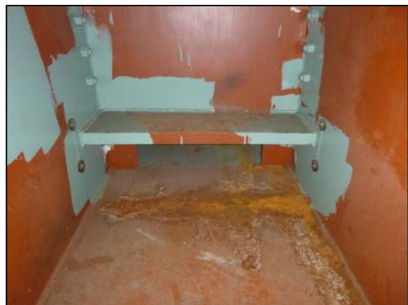
Photo 29: Bottom Flange, West of Girder D Diaphragm, Active Corrosion
