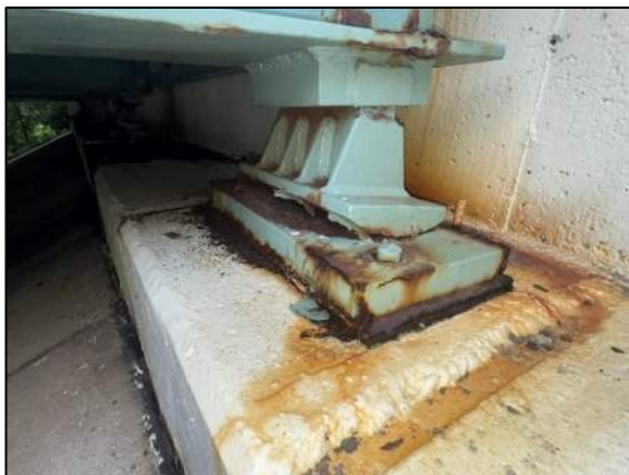
Photo 52: Poor Concrete Finish Behind Abutment 2 With Exposed Reinforcing Steel
