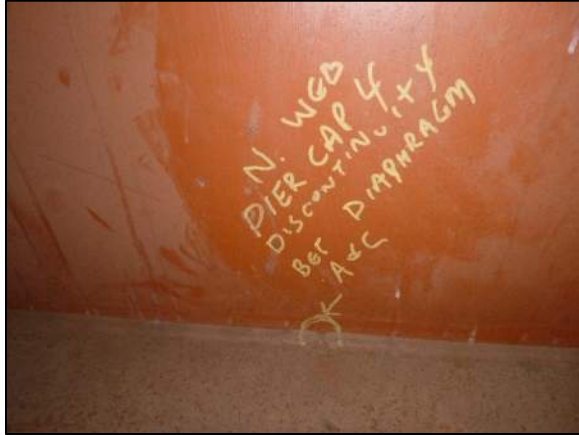
Photo 30: Discontinuity in Fillet Weld Between North Web and Bottom Flange Between Girder A and C Diaphragms
