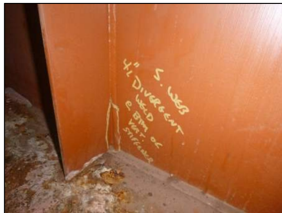
Photo 31: Divergent Fillet Weld in Interface of South Web and Vertical Web Stiffener, West of Girder D Diaphragm
