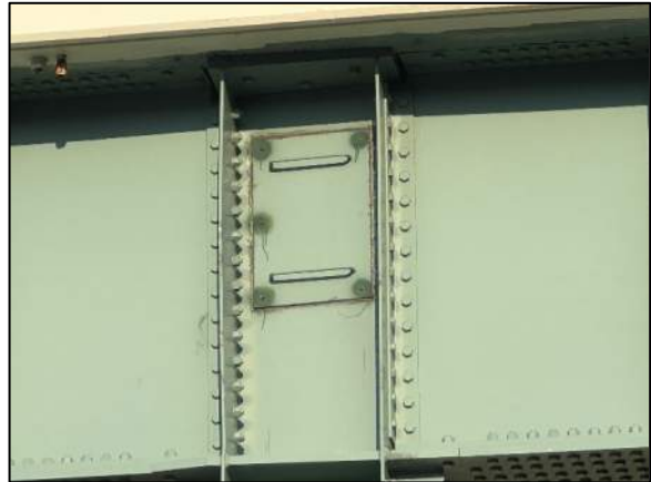
Photo 22: Missing bolt in West Access Hatch
