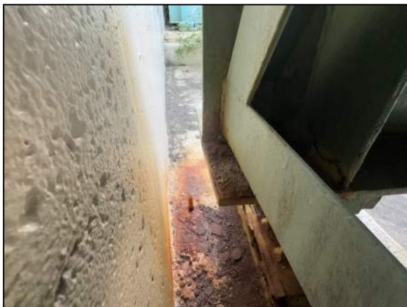
Photo 46: Section Loss on Girder G Lower Flange and Stiffener Behind Rocker Bearing at Abutment 2
