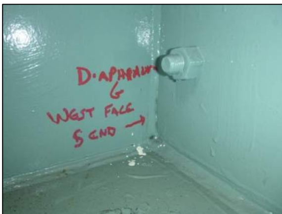
Photo 19: 3" Undercut in Fillet Weld Between Diaphragm and S Web
