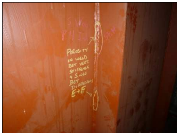
Photo 32: Fillet Weld Porosity Between South Web and Vertical Web Stiffener Between Girder E and F Diaphragms
