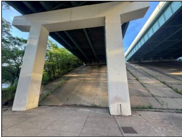
Photo 60: Abutment 2 Slope Protection Vegetation Growing Through Joints
