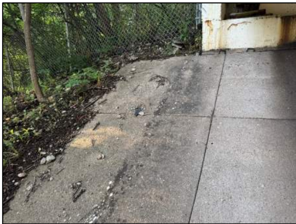
Photo 61: Settlement of Slope Protection at Abutment 2
