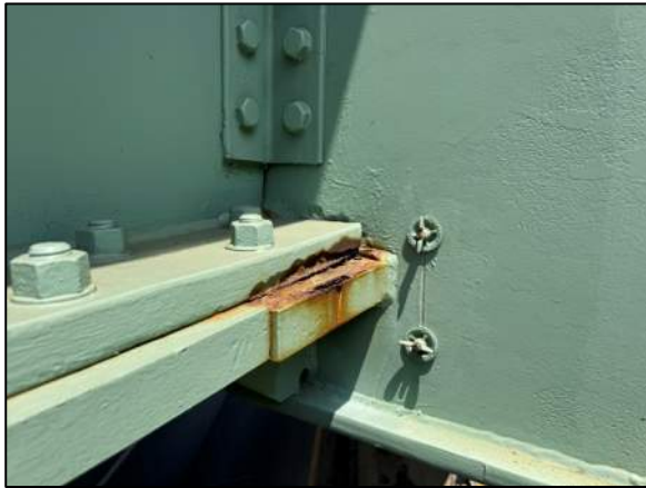
Photo 13: Active rust at Girder G, east face
