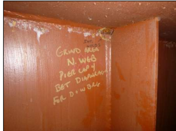
Photo 33: Unpainted Ground Area at Fillet Weld Intersection Between Girder D and West Bearing Stiffener
