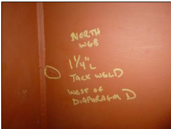
Photo 18: 1 1/4" L Tack Weld West of Diaphragm D, North Web
