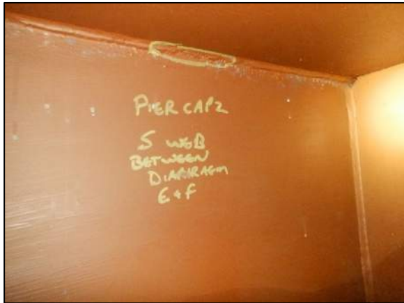
Photo 3: Weld Porosity in South Web Between Diaphragm E and F
