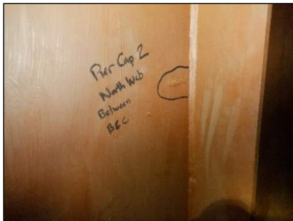
Photo 5: N Web Remaining Tack Welds Between Girder A and B
