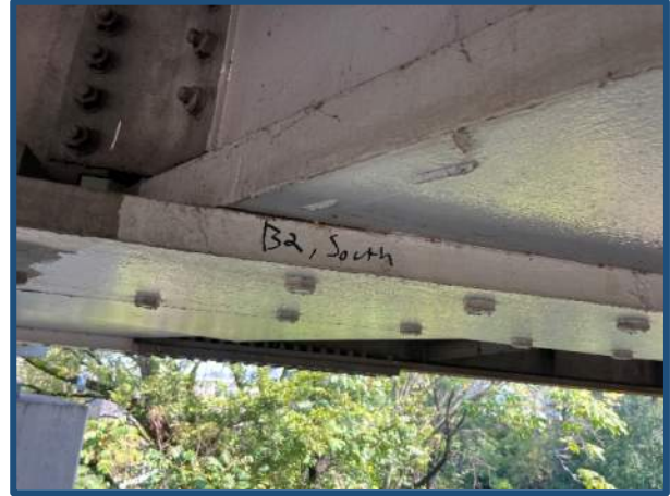
Photo 13: Tack welds on the west side of the bottom flange of the Pier Cap at Girder 2
