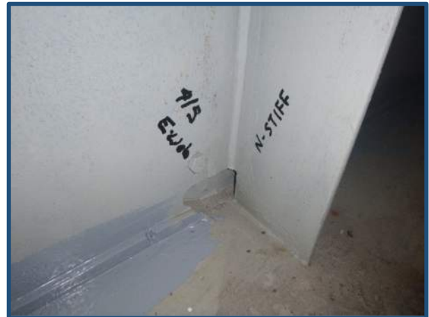
Photo 8: Un-welded butt joint between backer bar sections on the east web between Girder 4 and Girder 5
