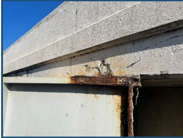
Photo 11: Minor corrosion on the south end of top flange at the bridge deck edge
