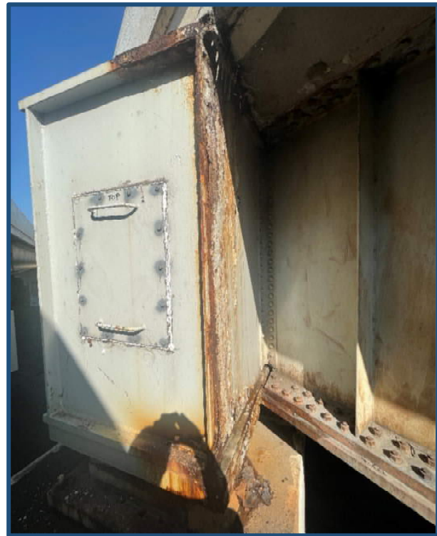
Photo 10: Surface corrosion on the south end of the Pier Cap
