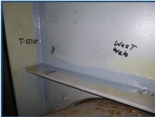
Photo 5: Triaxial weld between the transverse and longitudinal stiffeners at the water main
