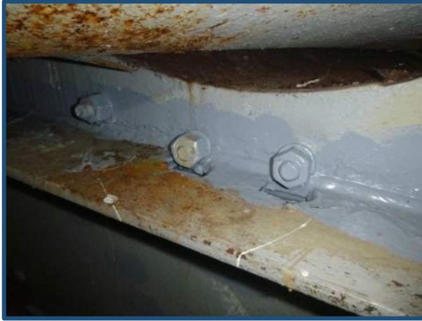
Photo 4: Thin welds at the water main bolted connection with the Pier Cap web
