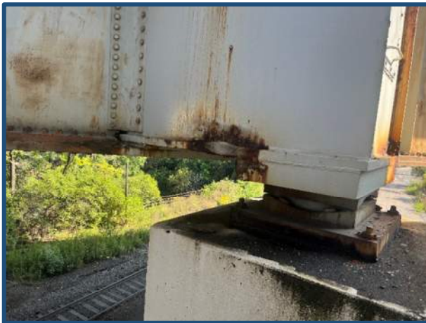
Photo 12: Pack rust at the west web of the Pier Cap at the Girder 6 connection
