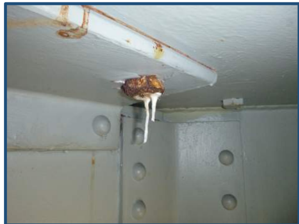
Photo 2: Evidence of leakage through the top flange at Girder 6
