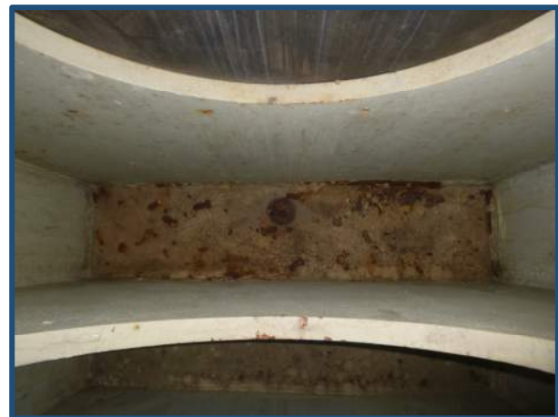
Photo 3: Surface corrosion on the north end of the Pier Cap bottom flange
