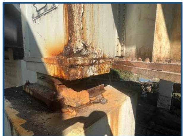
Photo 15: Surface corrosion and pack rust on the anchor bolts of the south bearing
