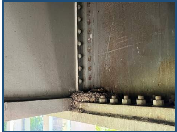
Photo 9: Typical bird debris buildup at the Girder connections with the Pier Cap
