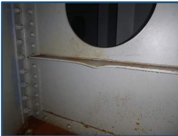
Photo 6: Bends in both horizontal stiffeners at the Girder 6 diaphragm
