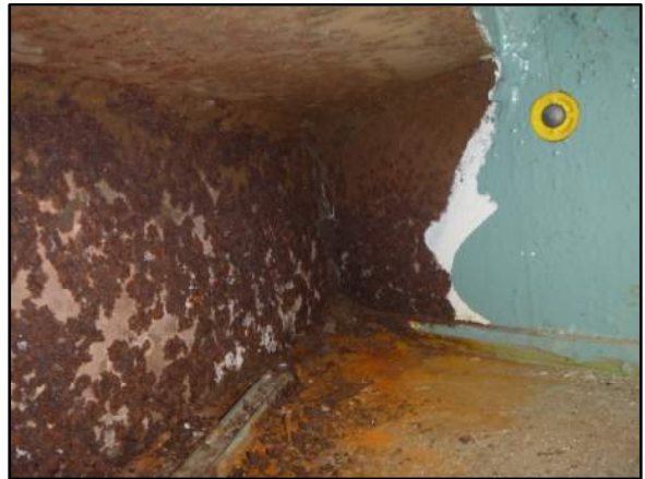
Photo 2: Active Corrosion Under Stiffener at Girder T, South Face
