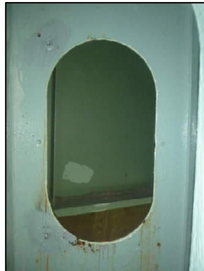
Photo 7: 1" of 100% Section Loss at South End Hatch Opening.
