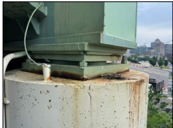
Photo 8: Typical Condition of North Bearing.
