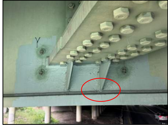
Photo 6: Typical Fillet Weld of the Girder Knee Brace and West Web Intersecting the Groove Weld Between the Web and Bottom Flange. Dog Bone Retrofit in Cap Web.
