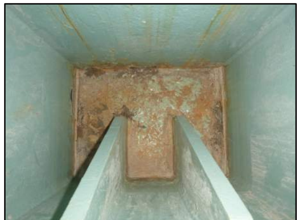
Photo 4: Surface Corrosion on the Bottom Flange Between the South Bearing Stiffener and End Plate.
