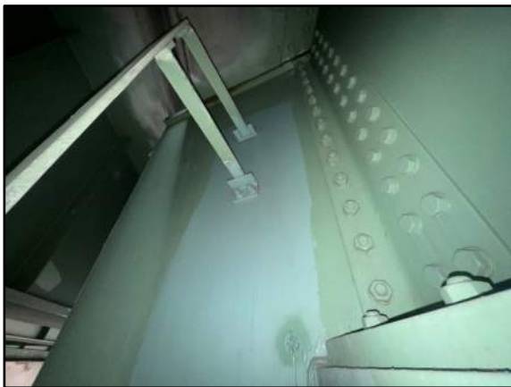
Photo 5: Bolted Downspout Brackets.
