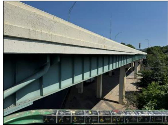
Photo 29: Typical View of Rail Cracking
