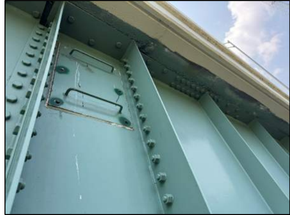
Photo 23: West Hatch, Left and Right top bolts have been sealed over
