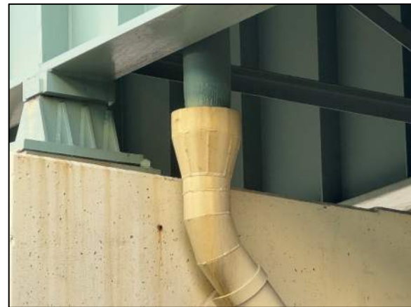
Photo 30: Typical Condition of Downspout to Bell Connection at Pier 5
