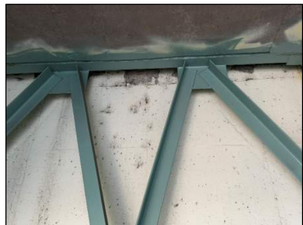
Photo 45: Poor Consolidation and up to 1" D Voids in Abutment 1 Backwall
