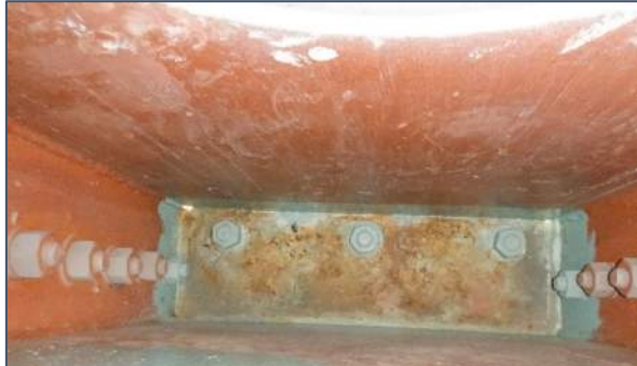
Photo 15: Reactivating Corrosion Along Lower Flange at Cap Ends
