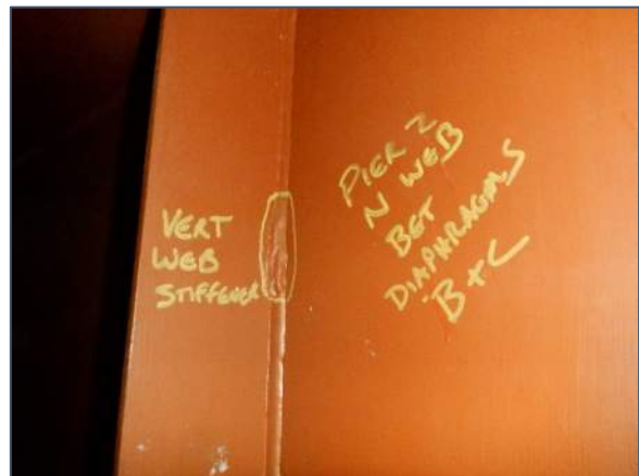
Photo 13: Multiple Weld Passes Between Web Stiffener and North Web Between Girder B and C
