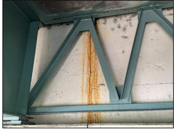
Photo 47: Rust Staining on Abutment 2 Backwall between Girder C and D
