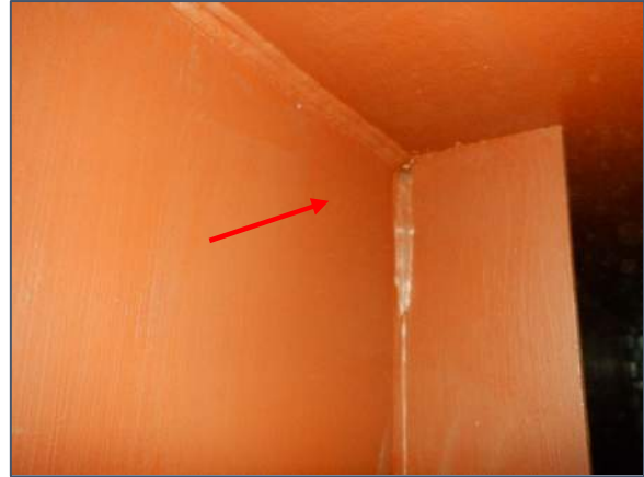
Photo 12: Ineffective Weld Cope Between Web Stiffener and Web Plates
