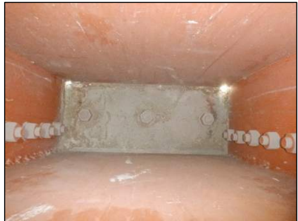
Photo 8: Typical Pitting in Bottom Flange Between Diaphragm and End Cap Openings
