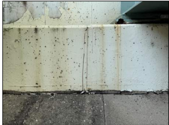
Photo 53: Up to 1" Settlement Along Full Length of Abutment Stem
