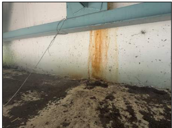
Photo 36: Typical Debris Build Up at Abutment 1; Girder A
