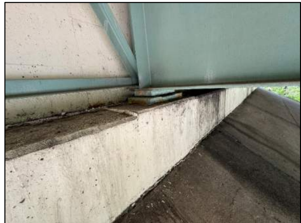
Photo 41: Typical Poor Consolidation Along Back of Seat at Abutment 2
