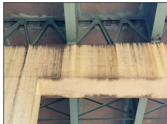
Photo 31: Full Length Staining of Pier 4 Underneath Deck Joint
