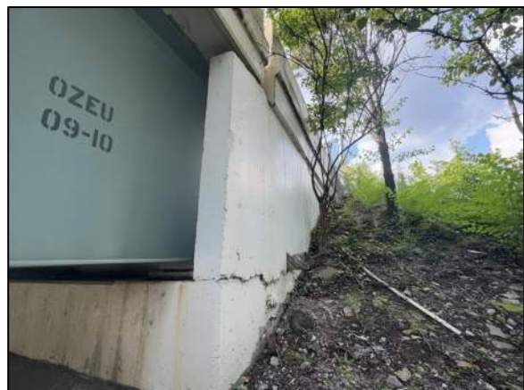
Photo 49: Abutment 2 NE Wingwall; Rough Transition to Cheek Wall
