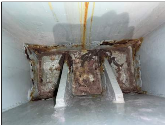
Photo 20: Active Rust Along Bottom Flange Between East Access Hatch and East Bearing Diaphragm
