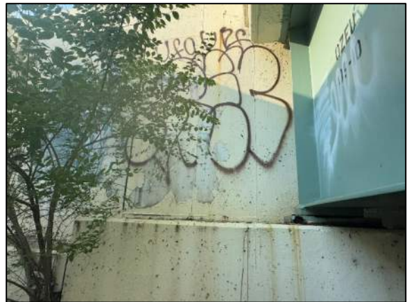
Photo 48: Missing Sealant and Graffiti on Abutment 2 North West Wingwall
