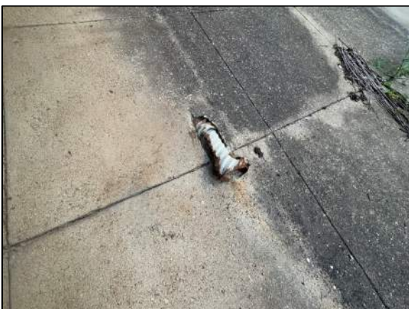
Photo 52: Typical Section Loss in Drainpipes in Slope Protection at Abutment 2.
