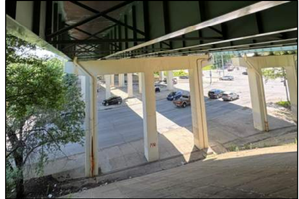
Photo 43: Minor Staining on Pier 6
