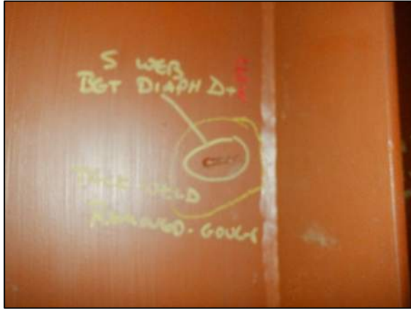
Photo 4: Gouge in South Web Between Girder D and C from Tack Weld Removal
