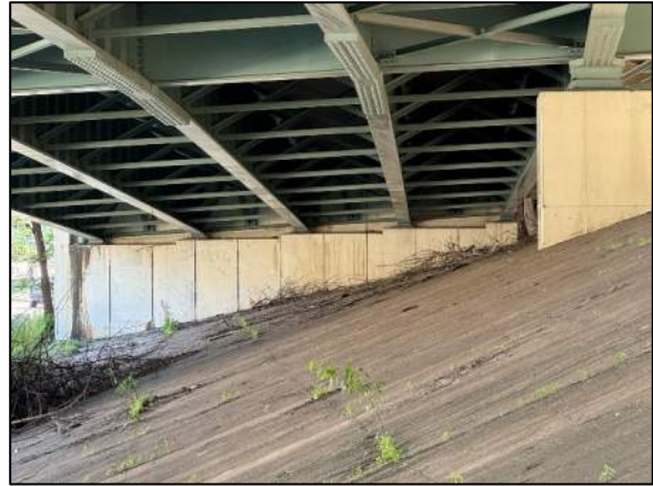
Photo 39: Drainpipe on East End of Abutment 1; Staining on Vertical Face of Stem
