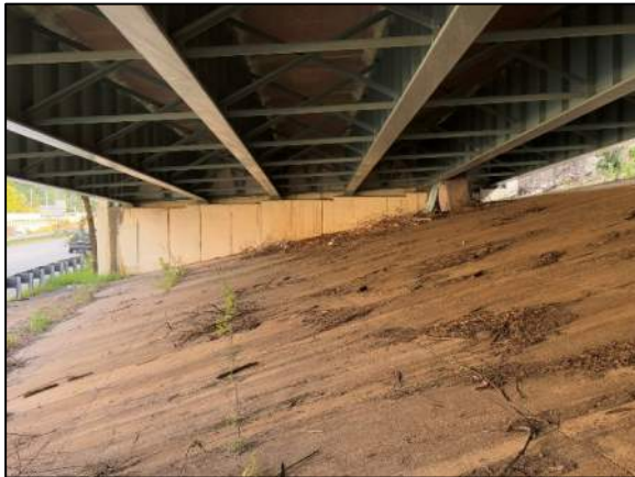
Photo 50: Debris Along Slope Protection Next to Pier 1
