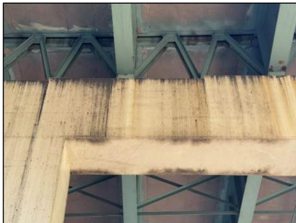
Photo 42: Moderate Staining Along Pier 4
