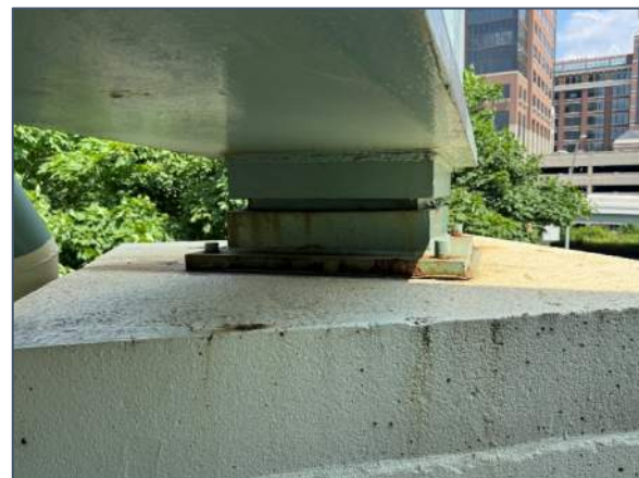
Photo 18: Typical Pot Bearing; Missing Nuts from Anchor Bolts
