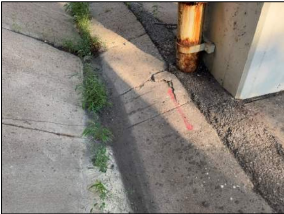
Photo 51: Cracked and Broken Slope Protection at Bottom next to Pier Column
