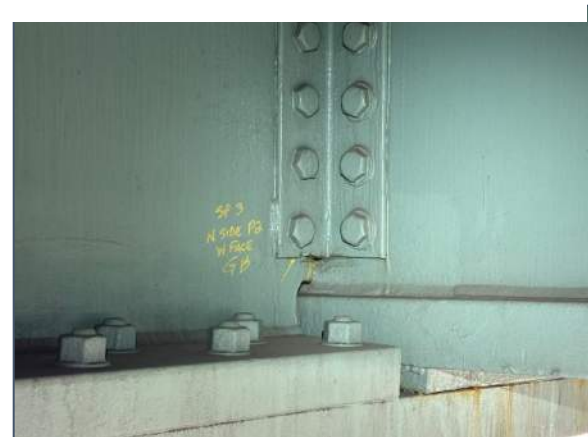
Photo 17: Tack Welds Ground but Not Removed at the West Face of Girder B and North Web
