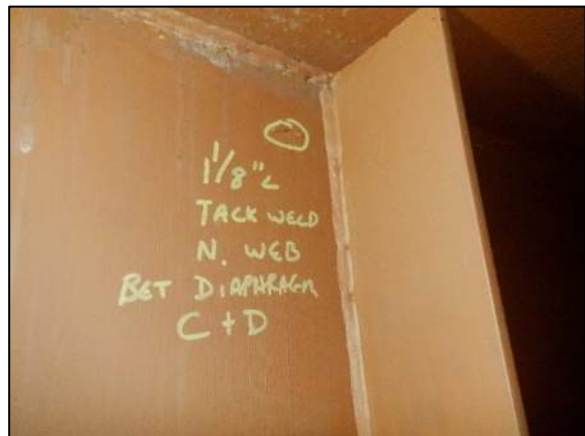
Photo 3: 1-1/8" Tack Weld on North Web Between Girder C and D
