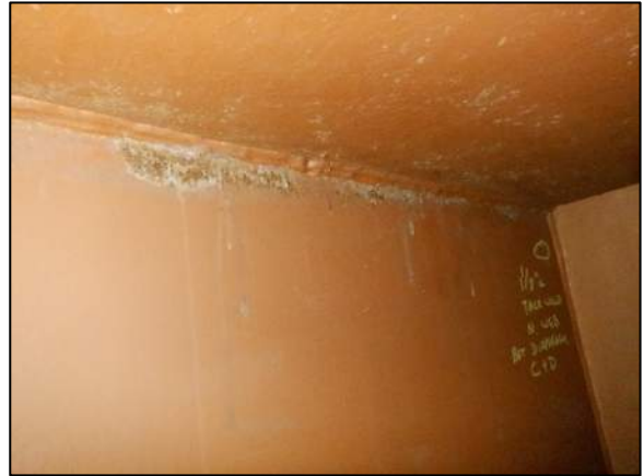
Photo 7: Typical Corrosion Along Upper Flange and Top of Webs Near Web Flange Interface
