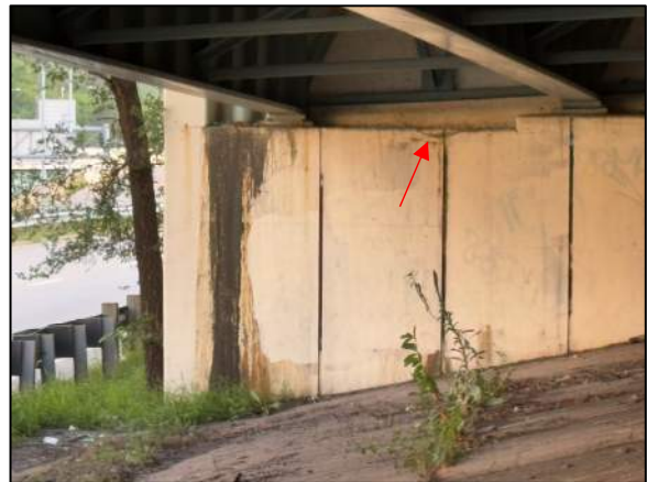
Photo 40: Abutment 1 Stem in Bay 5; 4' L X 1/4" W Crack and Delamination with Rust Staining
