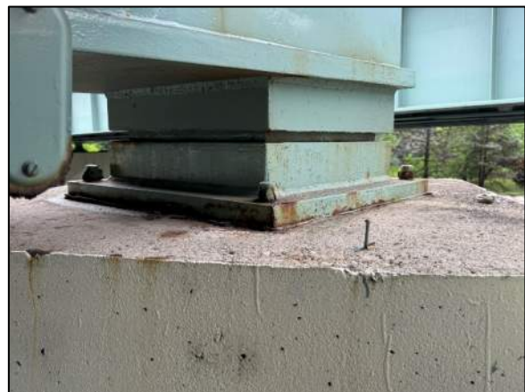
Photo 37: Minor Pitting and Corrosion on West Column Bearing for Pier 3
