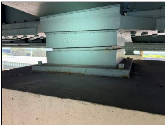
Photo 10: Nuts Missing from Anchor Bolts at Pot Bearings, Typical
