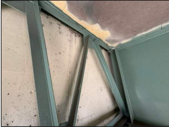
Photo 46: Typical View of Cracking in Backwall at Abutment 2
