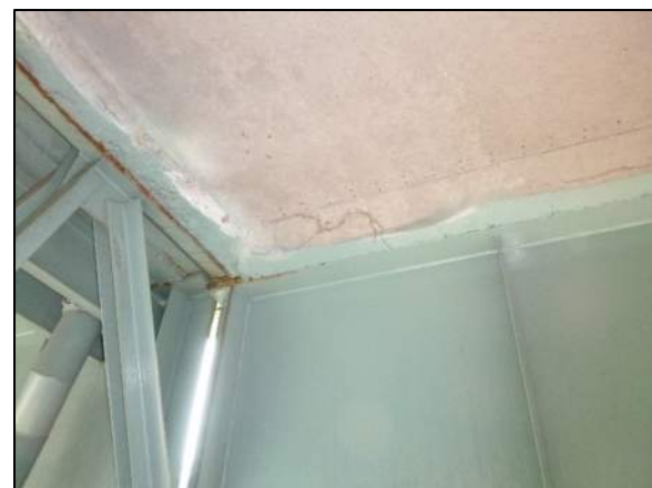
Photo 28: 3' L X Full Haunch Spall With 1' Delamination
