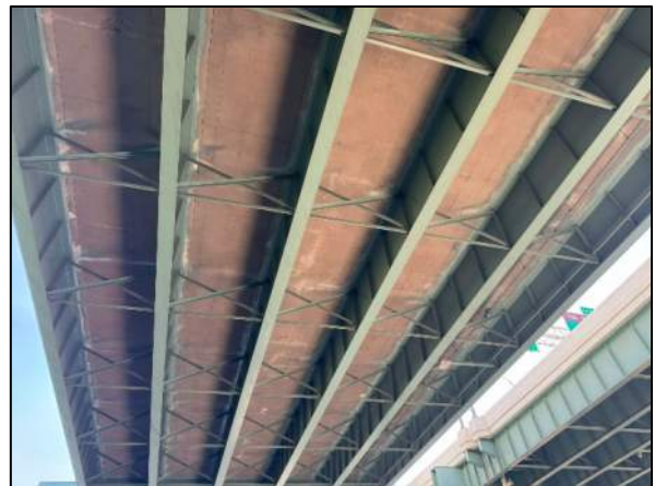
Photo 27: Efflorescence and Cracking in Span 5
