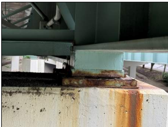
Photo 38: Peeling Paint and Active Corrosion on Sliding Bearings at Pier 4
