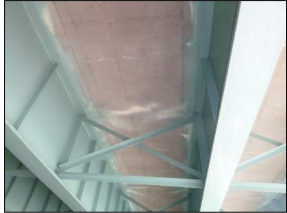
Photo 26: Underside of Deck in Bay 3, Span 2, Near Pier 2, Cracks with Efflorescence
