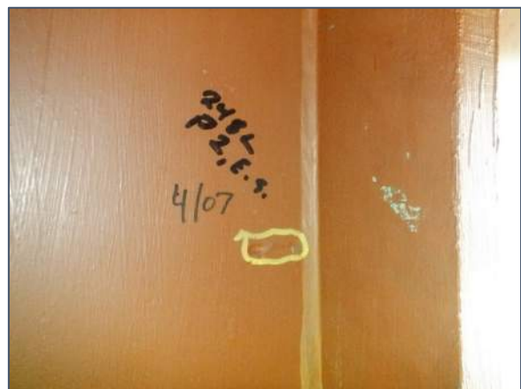
Photo 14: 1/2" L Gouge in North Web, East of East Bearing Diaphragm
