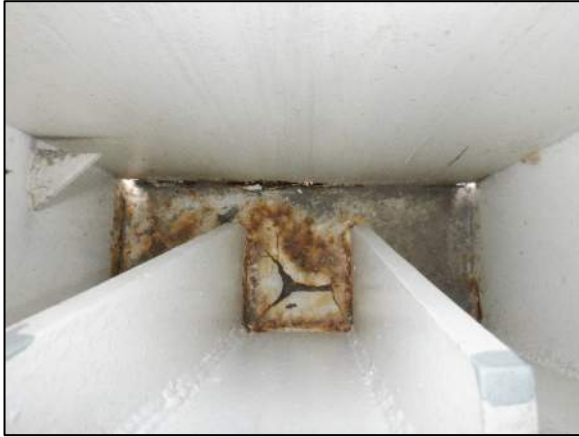
Photo 30: Peeling Paint and Active Corrosion Along Lower Flange Between Diaphragm and East Access Hatch
