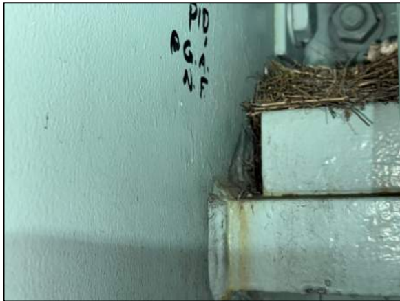
Photo 28: Section Loss on The North Web Behind Girder A. Minor Rust Staining and Bird Debris Present
