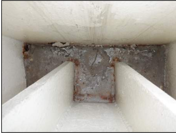
Photo 24: Active Corrosion and Paint Peeling Along Bottom of Web and Bottom Flange at West End Cap
