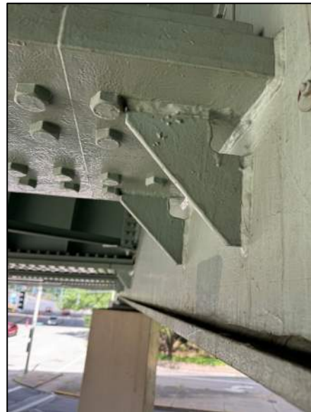
Photo 25: Typical Coped Knee Braces
