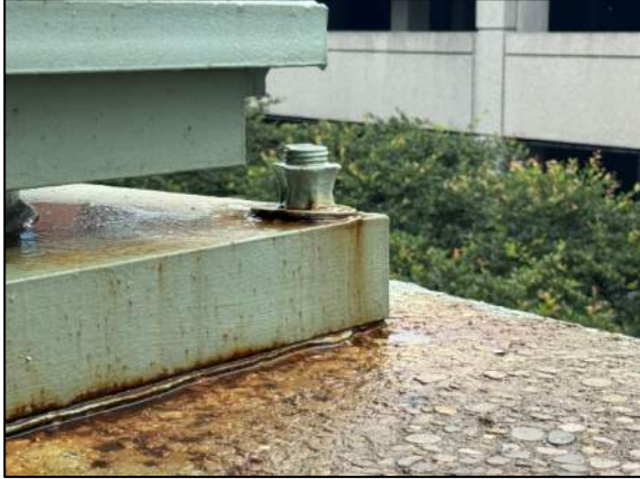
Photo 38: Up to 50% Section Loss of East Column, SE Anchor Nut. Section Loss Has Been Painted Over and Active Minor Surface Corrosion.
