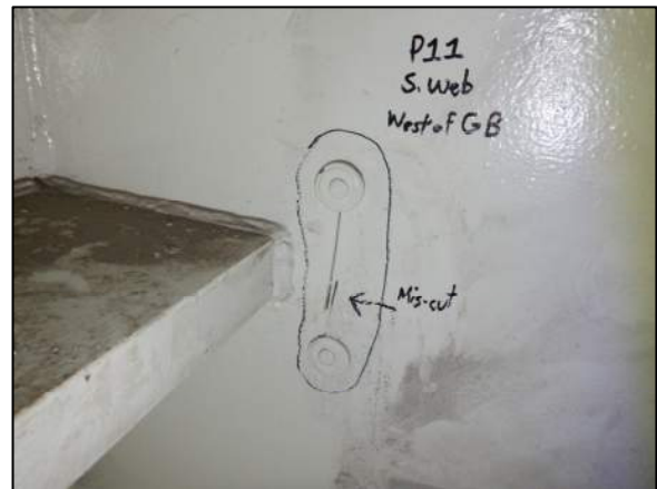
Photo 34: Mis-cut In Dog Bone Retrofit in South Web, West of Girder B
