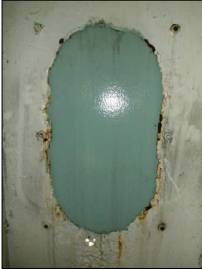
Photo 2: West Access Hatch Opening; Knife Edging and Corrosion Holes Along the Perforation in The End Diaphragm
