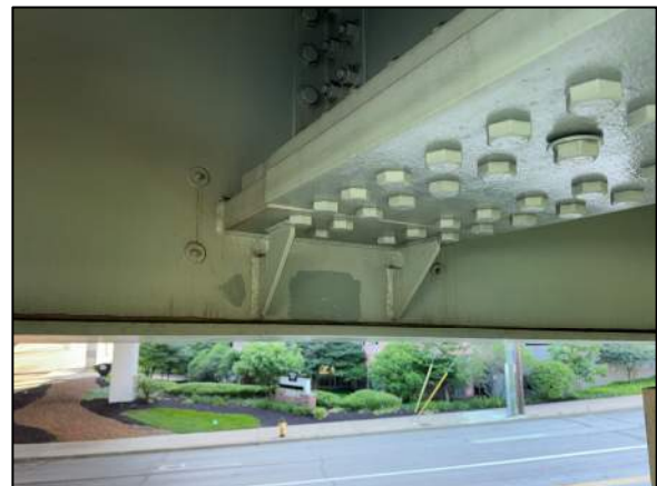
Photo 11: Retrofit Dog Bone Drilled Stress Relief Holes Connected with Saw Cut and Coped Knee Braces
