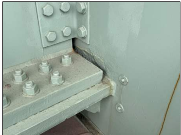
Photo 36: Section Loss in North Web Behind Bottom Flange of Girder A
