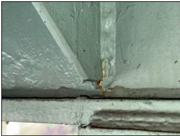
Photo 13: Paint Crack Located in Knee Brace Below Girder E
