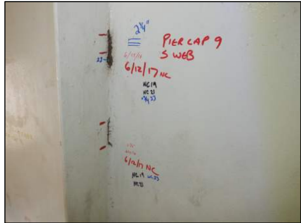
Photo 5: Girder J Diaphragm; 2-3/4" L and 1-1/2" Cracks in South Fillet Weld
