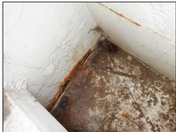
Photo 47: Typical Corrosion and Section Loss in Bottom Flange and Bottom of Web at West End Cap
