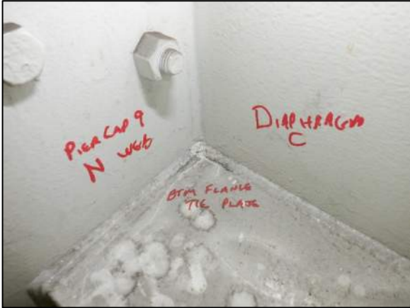
Photo 8: West Face of The Girder C Diaphragm, Tie Plate, and the North Web; Intersecting Welds Not Sufficiently Coped
