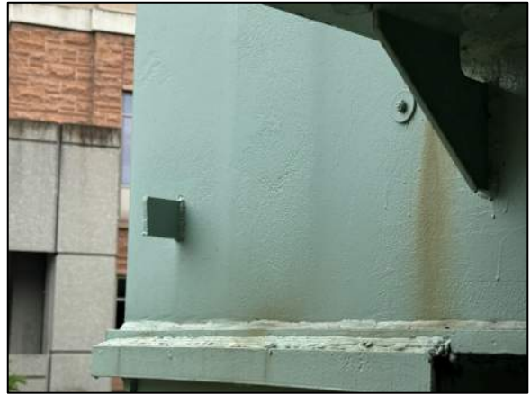
Photo 35: Remnants of Welded Drain Pipe Connection and Minor Surface Corrosion on North Web, East of Girder J
