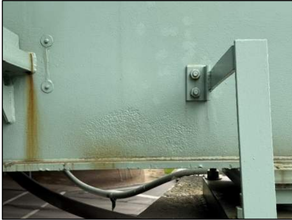
Photo 27: Minor Fretting Corrosion Between Bolted Connection on North Web and Lower Lateral Brace on West Side of Girder H
