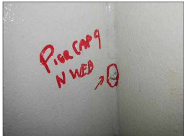
Photo 7: North Web at The Stiffener East of The Girder F Diaphragm; Irregular Weld
