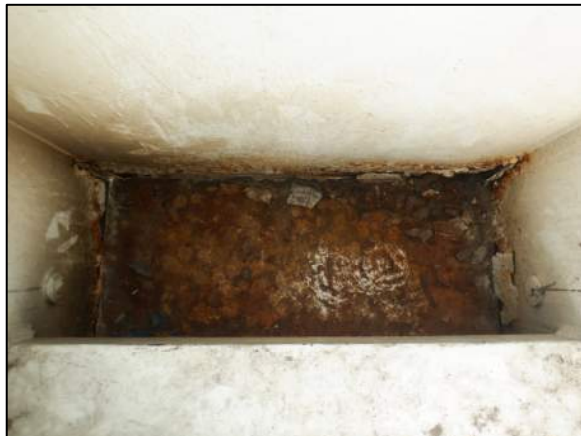
Photo 4: Bottom Flange Adjacent to East End; Painted Over Pitting and Reactivating Laminating Corrosion
