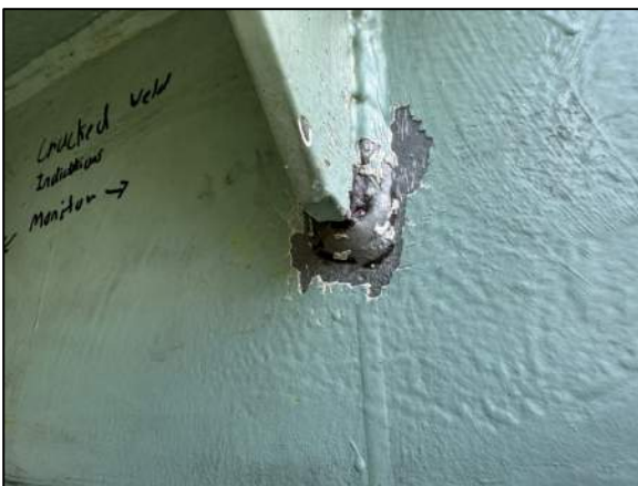
Photo 52: Cracked Weld Indications on East Knee Brace Fillet Weld
