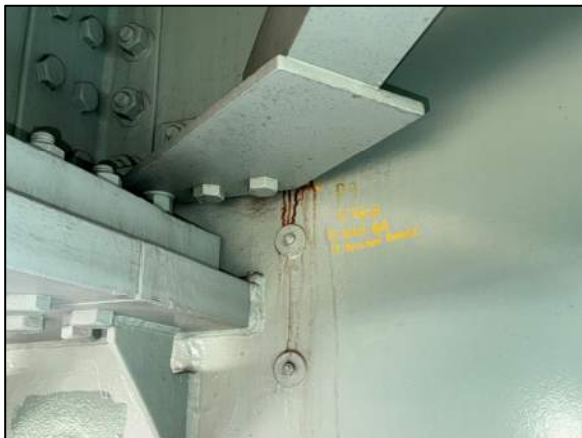
Photo 14: South Web East of Girder G; Corrosion Staining at Bolted Connection for Lower Lateral Bracing
