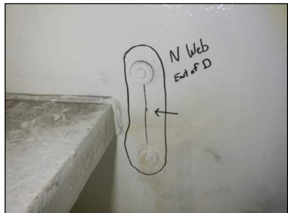
Photo 22: Mis-Cut Dog Bone Retrofit in North Web East of Girder D
