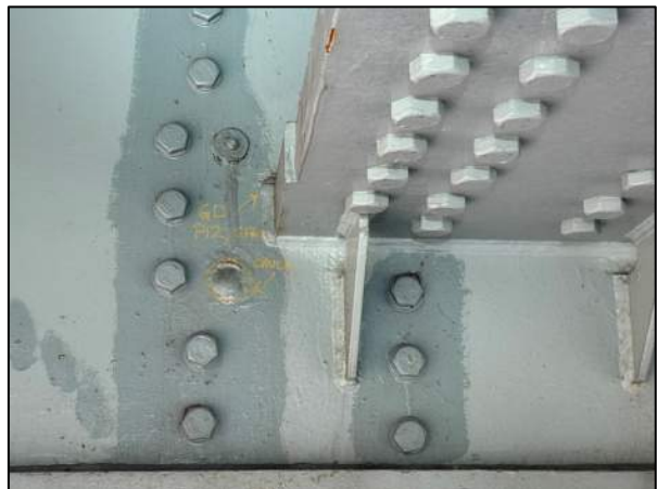
Photo 49: Missing Bolt in South Web, West of Girder D; Hole Filled with Caulk and Painted Over
