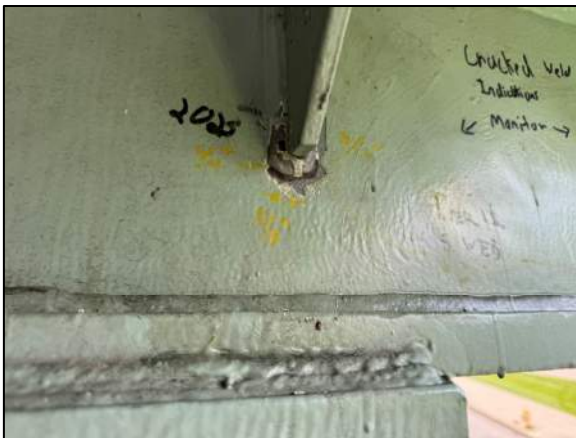
Photo 51: Cracked Weld Indications on West Knee Brace Fillet Weld
