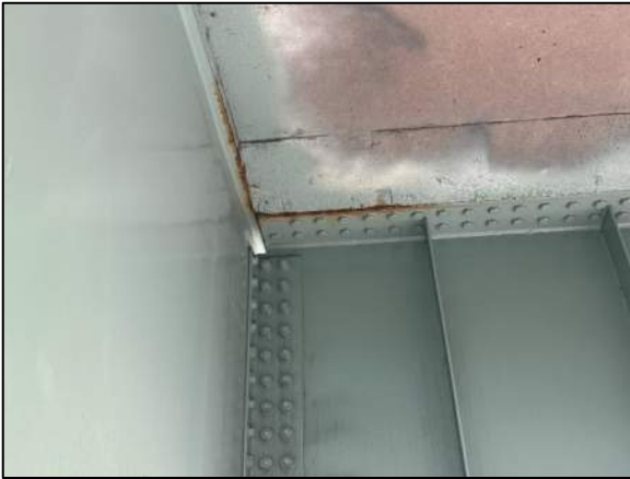
Photo 50: Rust Staining Along Top Flange of Pier Cap at Girder J
