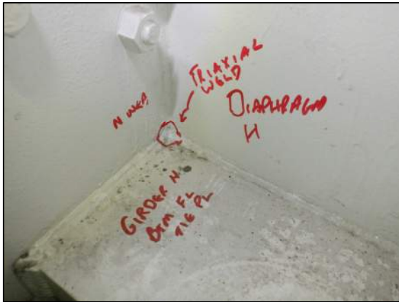
Photo 43: Triaxial Weld Between North Web, Diaphragm H, And Bottom Flange Tie Plate
