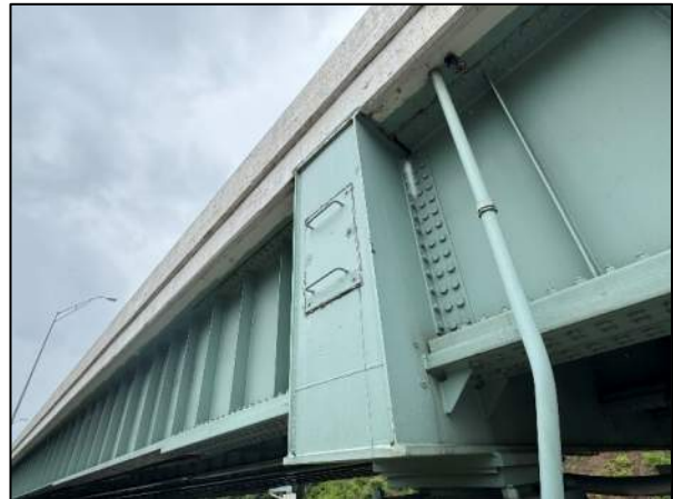
Photo 48: West Access Hatch; Middle Bolt Hole Filled with Caulk
