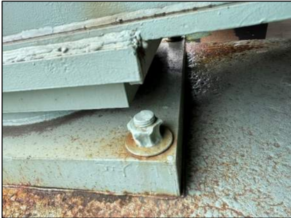
Photo 39: Up to 50% Section Loss of East Column, NW Anchor Nut. Section Loss Has Been Painted Over and Active Minor Surface Corrosion .
