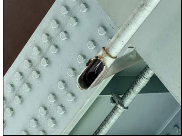
Photo 40: Missing Conduit Cover, North Side, East of Girder E.
