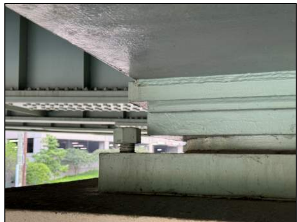
Photo 16: West Bearing Unseated Anchor Nut on Center Column
