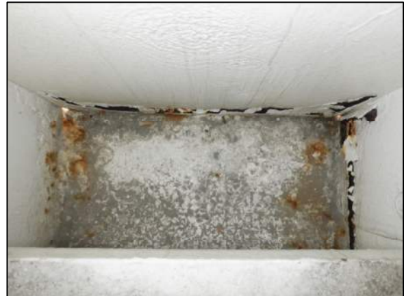
Photo 23: Moderate Pitting on Bottom Flange and Bottom of Webs Between Girder J and East End Plate
