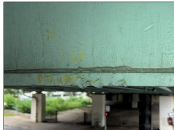
Photo 26: 4" X 1" Minor Impact Damage to North Side of Bottom Flange West of Girder B, no change.
