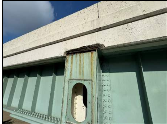
Photo 10: East End of Pier Cap; Active Corrosion on Top Flange and Corrosion Staining. Spall size unchanged.
