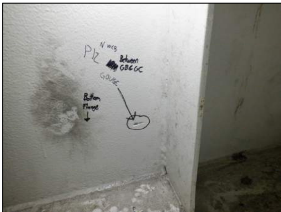
Photo 44: Gouge in North Web, Near Bottom Flange, Between Girder B and Girder C
