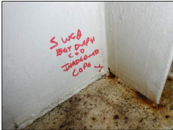
Photo 19: Insufficient Cope in South Web Between Diaphragm C and D
