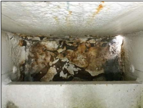
Photo 3: Bottom Flange Adjacent to West End; Painted Over Pitting and Reactivating Laminating Corrosion
