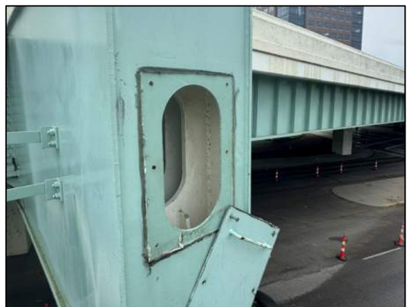
Photo 37: Painted Over Pitting on East Access Hatch
