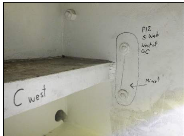
Photo 46: Mis-Cut Vertical Cut in South Web Dog Bone Retrofit, West of Girder C
