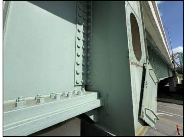
Photo 15: Pitting Along the Top of The Bottom Flange, Knee Brace, And Web
