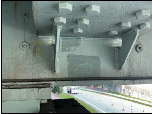
Photo 12: 2" L 3/16" D Gouge on North Web, At Girder B from Coping
