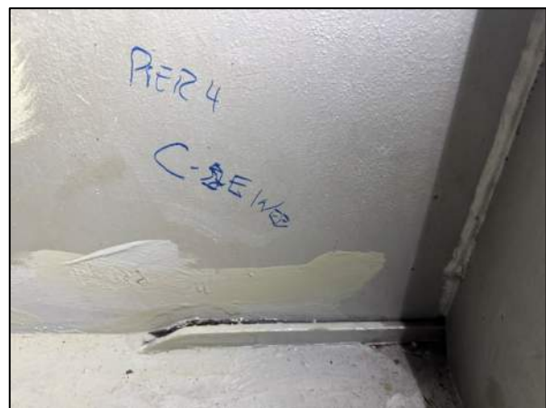
Photo 25: Backer bar pulling 1/2" away from the Pier Cap 4 web plate west of Girder 3.
