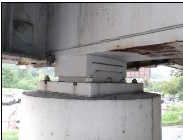
Photo 30: Minor surface corrosion on the masonry plate and anchor bolts at the Pier Cap 4 east bearing.
