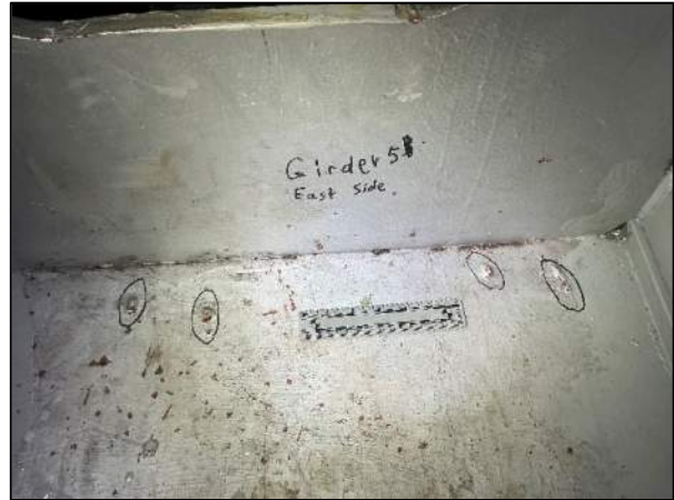
Photo 7: Four tack welds ranging from 1/2" to 1" on the bottom flange of Pier Cap 3 east of Girder 5.
