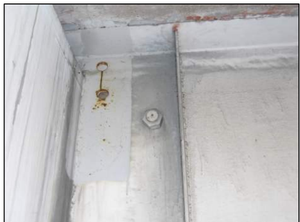
Photo 16: Typical view of errant sawcuts on the Girders.
