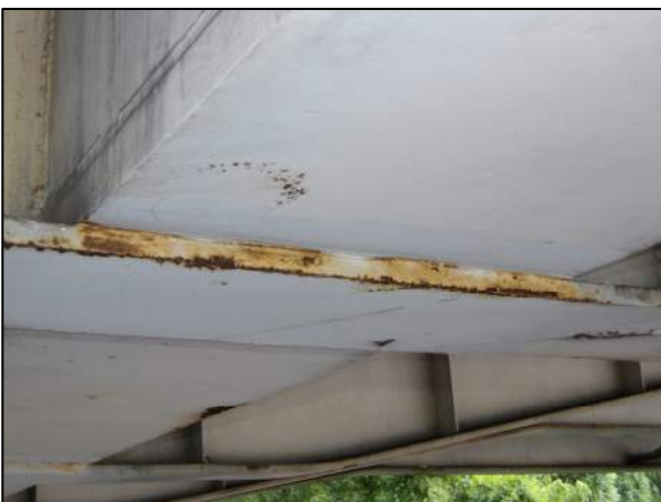
Photo 36: Typical gouges on the Pier Cap bottom flange from tack weld removal.
