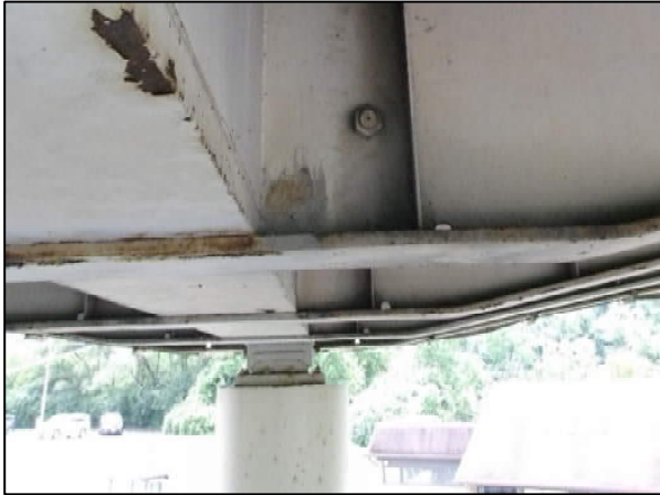
Photo 18: Gouges of the bottom flange of Pier Cap 3 at the west side of Girder 4 from stitch weld removal.
