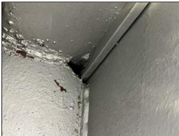
Photo 5: Cracked tack weld between the top flange and north web between the east bearing and Girder 7 at Pier Cap 3.
