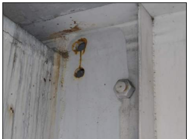
Photo 33: Typical gouges in the Girder sawcut retrofit.
