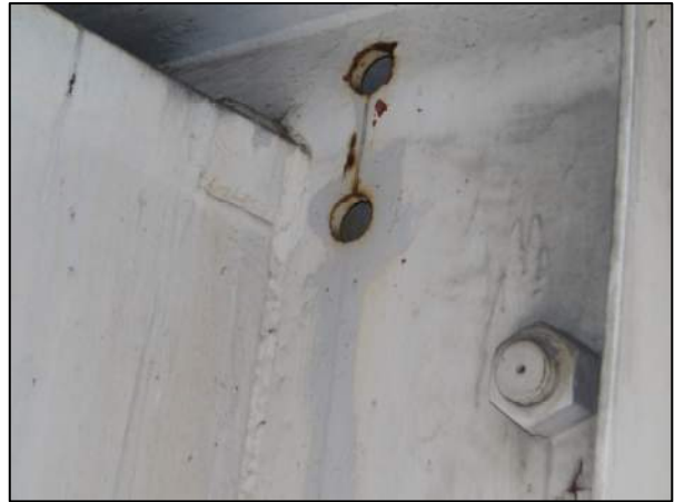
Photo 15: Typical gouges in the Girder sawcut retrofit.
