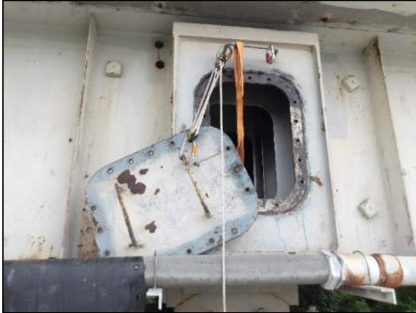
Photo 34: Typical condition of Pier Cap Door and Seal, east side.
