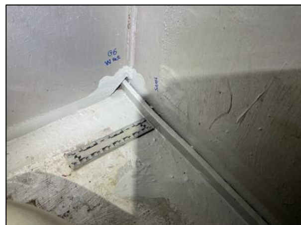
Photo 3: Gap between the backer bar and south web plate west of Girder 6 at Pier Cap 3.
