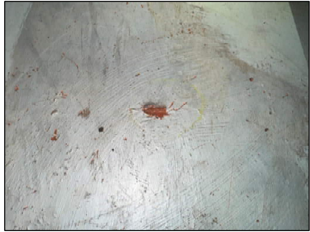
Photo 29: Partially ground tack weld west of Girder 5 on the bottom flange of Pier Cap 4.
