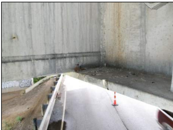
Photo 20: No change to the 1-1/2" combination sawcut and crack on the northeast corner of Girder 5 at the north face of Pier Cap 3.
