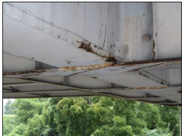
Photo 32: Impact damage with peeling paint and surface corrosion on the bottom flange at the north face of Pier Cap 4 and Girder 5.
