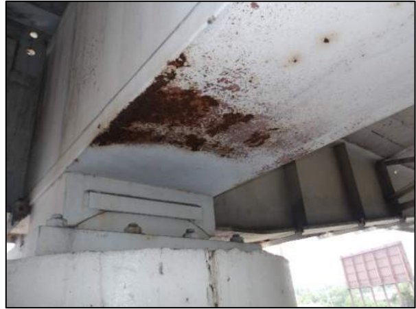
Photo 31: Typical minor surface corrosion on Pier Cap 4
