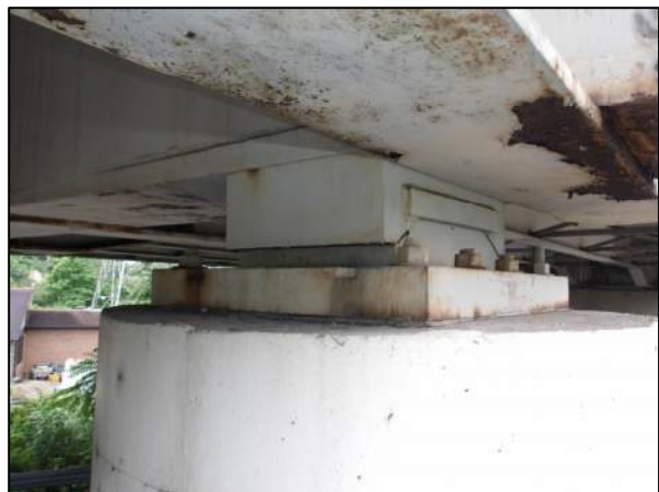
Photo 11: Minor surface corrosion on the masonry plate and anchor bolts at the Pier Cap 3 west bearings.
