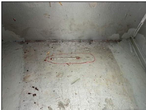
Photo 28: 7" transverse weld east of the Girder 6 diaphragm on the bottom flange of Pier Cap 4.
