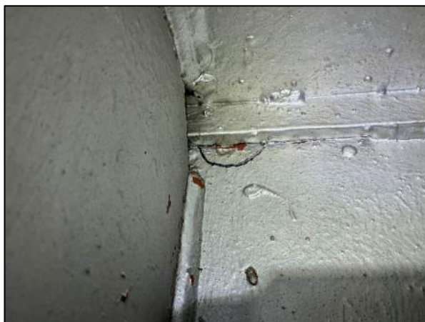
Photo 6: Cracked tack weld between the top flange and south web at Girder 7 at Pier Cap 3.
