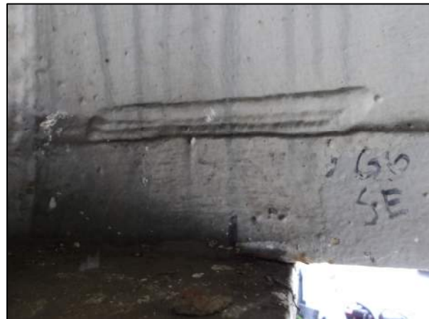
Photo 22: 1-1/2" combination sawcut and crack in the weld on the southeast corner of Girder 6 at the south face of Pier Cap 3.
