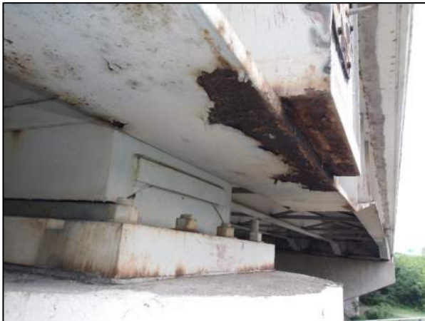
Photo 13: Up to 5/16" pack rust between the Girder 1 bottom flange and the pier cap at the west end of Pier Cap 3.
