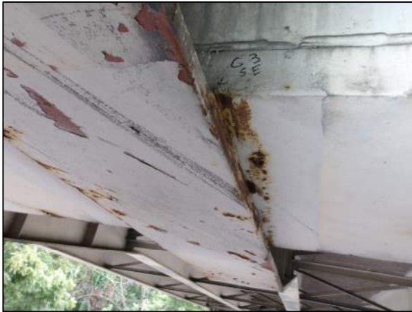
Photo 12: Minor freckling corrosion, peeling paint and vehicle scrapes on bottom flange.
