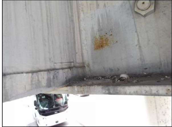
Photo 21: 3/4" sawcut and 1" crack on the northwest corner of Girder 4 at Pier Cap 3.
