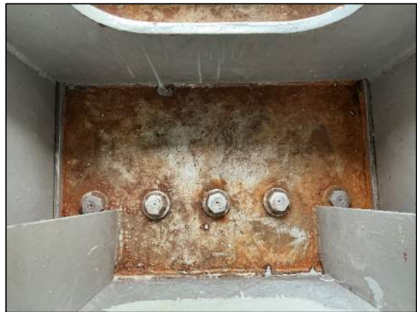
Photo 2: Surface corrosion on the bottom flange of Pier Cap 3 adjacent to west access hatch.
