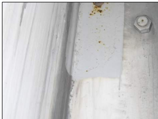
Photo 17: Typical overlapping welds on the Pier Cap 3 web plates.
