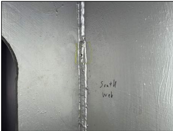
Photo 27: Poor quality welds displaying overlapping and porosity on the diaphragms of Pier Cap 4.
