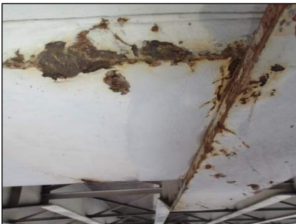
Photo 14: 4" long area of impact damage on Pier Cap 3 bottom flange west of Girder 3.
