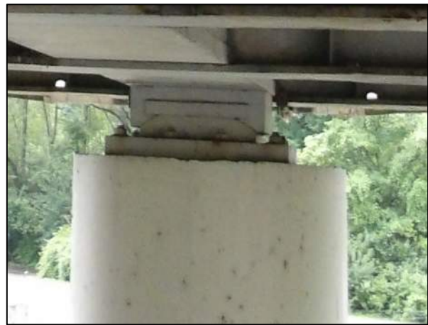
Photo 10: Typical Peeling Paint and surface corrosion at the east bearing of Pier Cap 3
