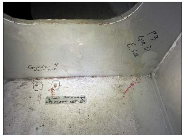
Photo 8: Additional 1/2" tack welds on the bottom flange east of Girder 4.
