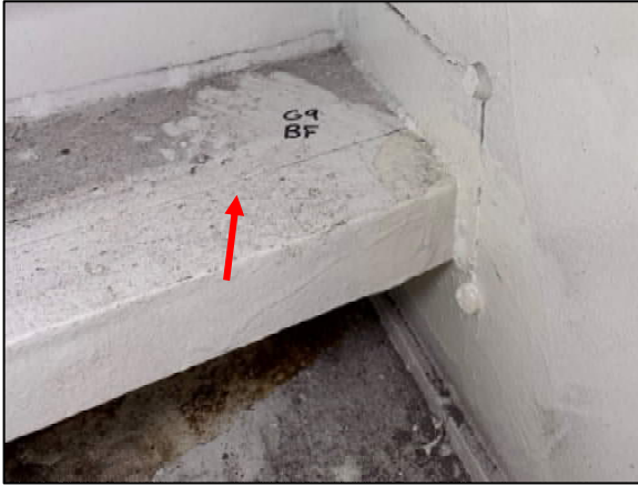
Photo 62: 20" long (1/16" deep) cut in the bottom flange strap plate of Girder 9
