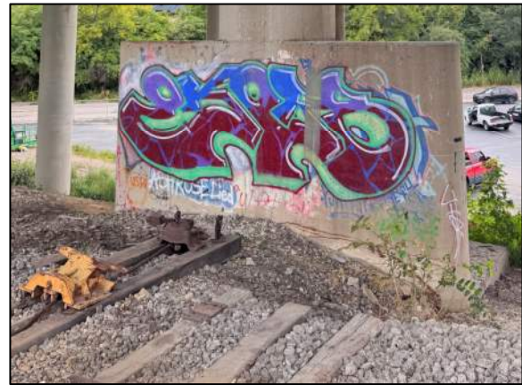
Photo 17: Erosion at the base of the north column
