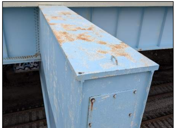
Photo 28: Fading paint and surface corrosion on the top flange between Girder 10 and the south end of Pier Cap 5
