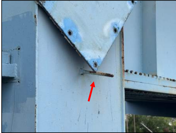
Photo 57: 8" long steel rod and nut welded to the pier cap below north access hatch
