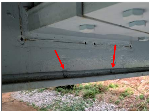
Photo 70: Remnants of knee braces and fillet welds, typical at all girders
