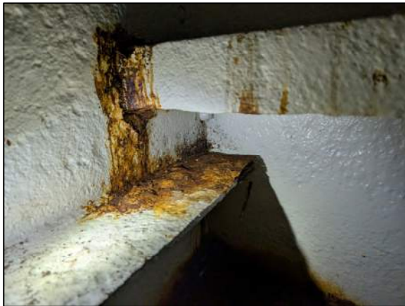
Photo 3: Painted over pitting on web plate on the south side of Girder 6
