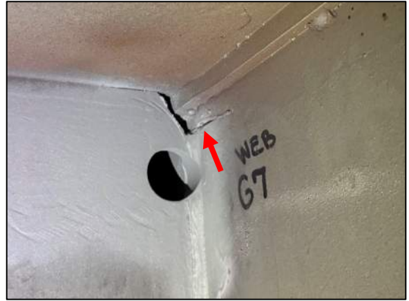
Photo 24: 1-1/2" gouge in east web on the south side of Girder 7
