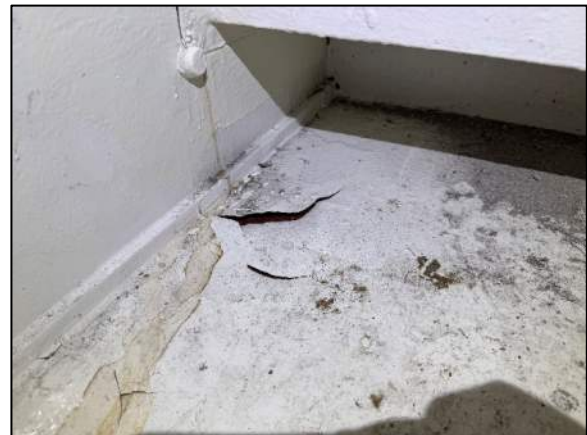
Photo 60: Typical scattered minor areas of peeling paint on the interior
