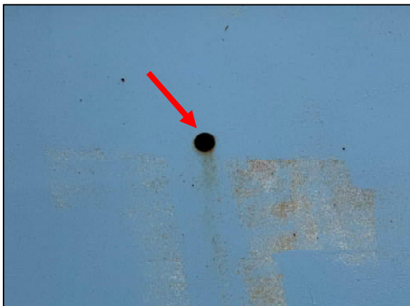
Photo 15: Missing expansion plug in the west web retrofit hole south of Girder 10
