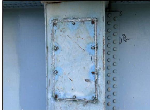
Photo 41: Areas of missing paint and surface corrosion at the north end
