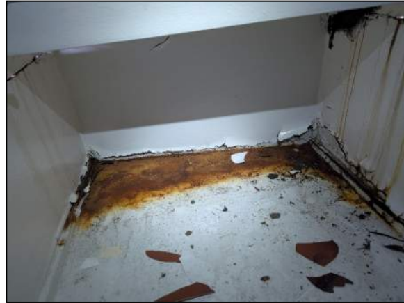
Photo 5: Peeling paint and active corrosion resulting from leakage through the retrofit on the south side of Girder 10
