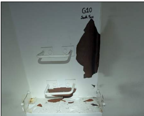
Photo 4: Paint loss on the south face of the Girder 10 diaphragm
