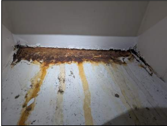
Photo 2: Signs of water with active corrosion and bubbling paint on the south side of Girder 9A
