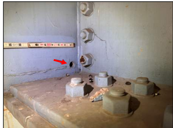
Photo 79: Missing expansion plug on the west web retrofit at Girder 5
