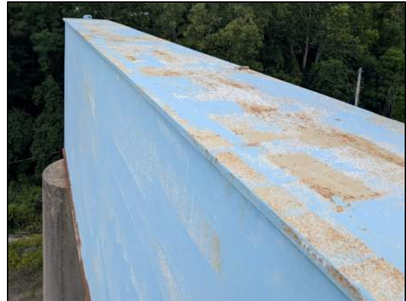
Photo 65: Typical fading paint condition on exterior, exposed southern end of pier cap shown
