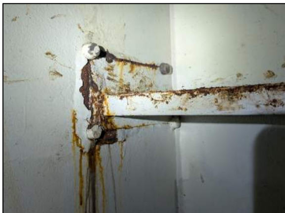
Photo 40: Typical leakage, bubbling paint, and surface corrosion due to missing epoxy sealant at Girder 6 retrofit
