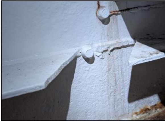
Photo 8: Typical incomplete longitudinal stiffener removal between Girders 7 and 8
