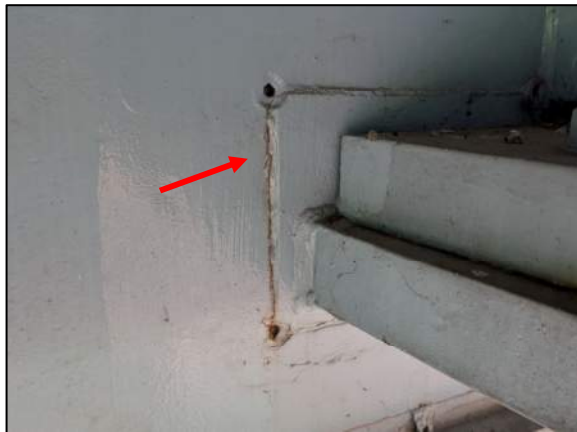
Photo 69: 1/16" bowing of the east web retrofit on the south side of Girder 6
