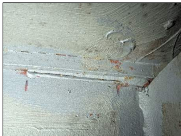
Photo 73: 2" remaining of a partially ground fillet weld between the east web and top flange between Girders 2 and 3
