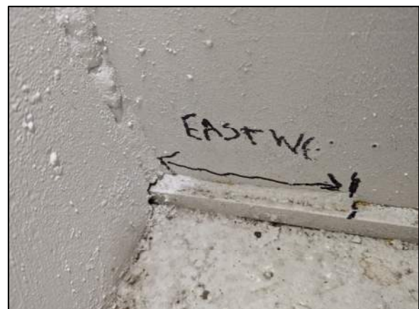
Photo 52: 5-1/2" long fillet weld at bottom flange between south bearing diaphragm and south end plate.
