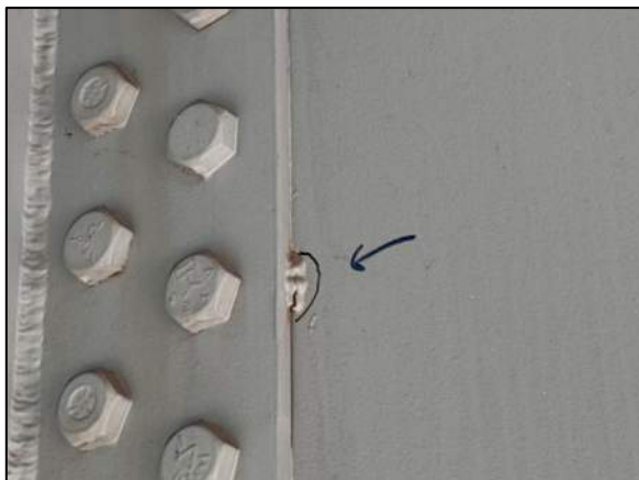
Photo 46: Cracked tack weld on the Girder 4 and pier cap west web plate connection
