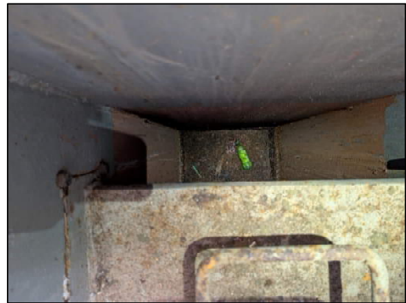
Photo 36: Area of laminating corrosion on bottom flange between Girder 1 and the north end of the cap
