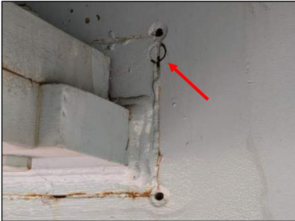
Photo 68: Miss-drilled retrofit hole in the west web at Girder 5
