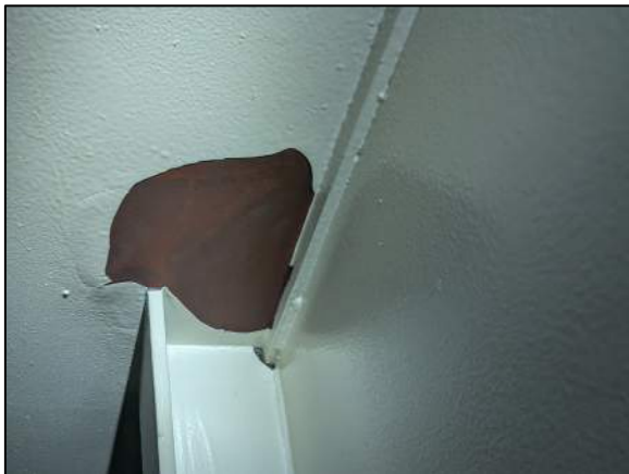
Photo 49: Typical scattered peeling paint throughout the interior of the pier cap
