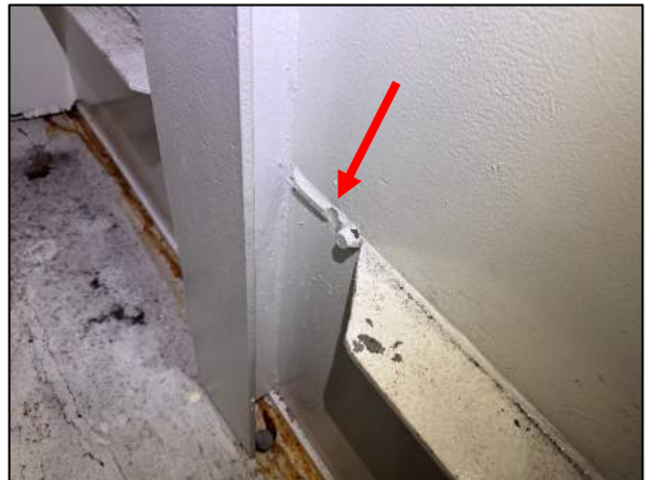
Photo 26: Incomplete removal of longitudinal stiffener between Girder 6 and 7
