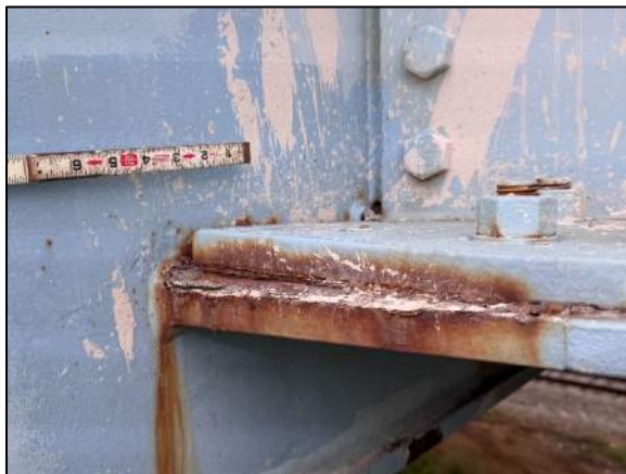
Photo 76: Corrosion reactivating at a location of painted over section loss on west web at Girder 1
