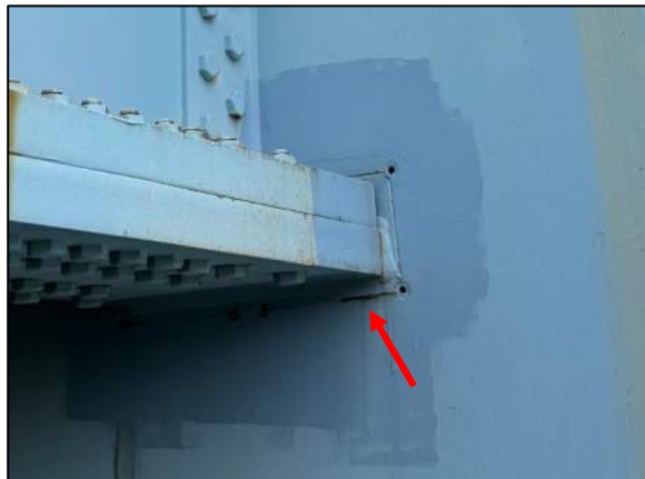
Photo 58: Missing epoxy sealant east web retrofit on the south side of Girder 10
