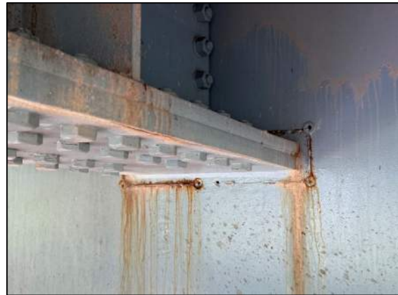
Photo 42: Corrosion is beginning to reactivate at previously painted over section loss at Girder 6 and pier cap east web plate
