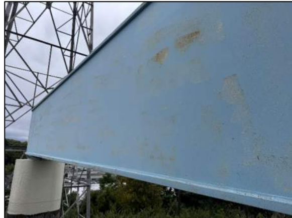
Photo 10: Typical fading paint and surface corrosion at the south end of the pier cap
