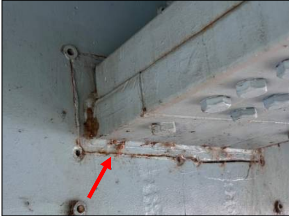
Photo 13: Thin cracks in epoxy with rust staining on east web retrofit at Girder 7
