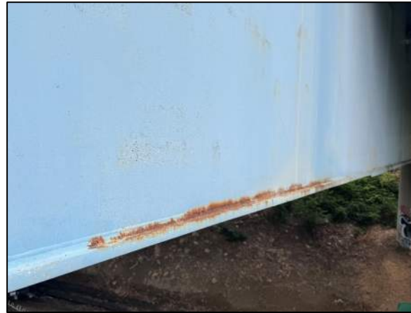
Photo 54: Typical fading paint and surface corrosion at the south end
