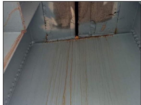
Photo 78: Corrosion and rust staining from leakage through deck joint between Girders 5 and 6
