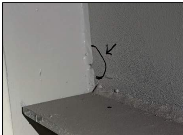
Photo 53: 1-1/4" discontinuity in the transverse stiffener weld on west web between Girders 7 and 8
