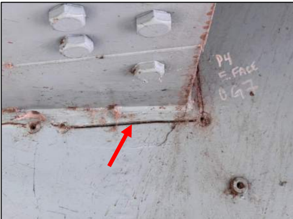
Photo 14: Missing epoxy on the east web retrofit at Girder 7
