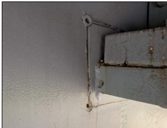
Photo 31: Retrofit in west web deflected up to 1/4" at Girder 6
