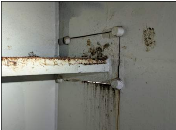
Photo 39: Typical leakage, bubbling paint, and surface corrosion due to missing epoxy sealant at Girder 7 retrofit
