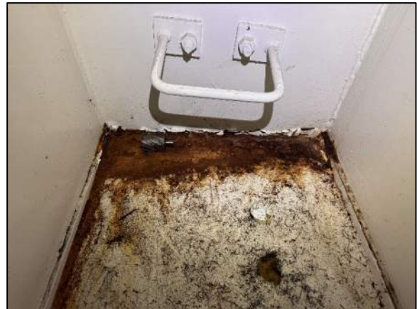
Photo 19: Evidence of ponding with corrosion on the bottom flange on the south side of Girder 5
