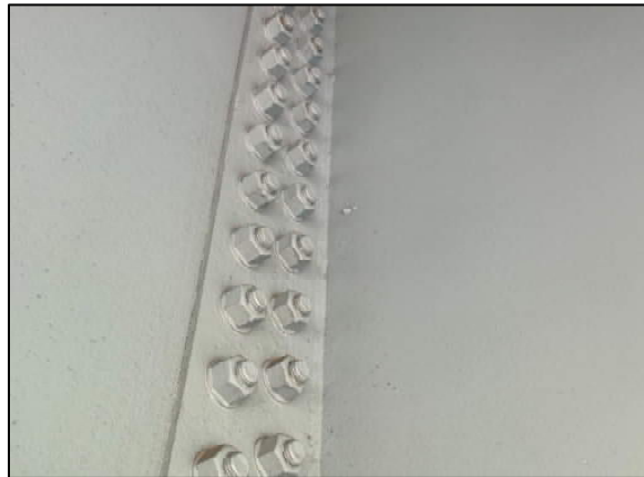
Photo 11: 3/4" tack weld on the west web at the south face of Girder 6
