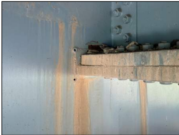
Photo 45: East web retrofit at Girder 5 bowing inward approximately 1/8"
