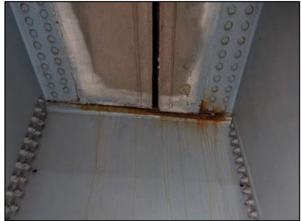
Photo 27: Corrosion and rust staining on top flange and web between Girders 5 and 6.
