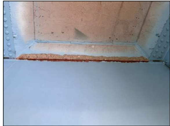
Photo 77: Typical corrosion on top flange between Girders on the east and west web
