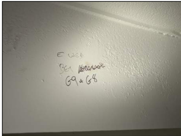
Photo 6: Inadequate surface preparation leading to bubbling paint on web plate between Girders 8 and 9
