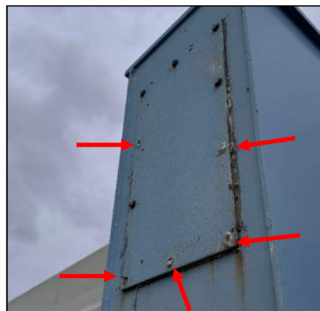
Photo 43: Five missing bolts on south hatch
