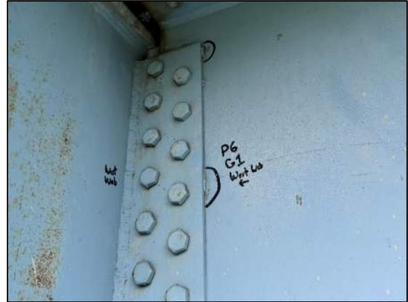
Photo 47: one cracked tack weld and one poor quality tack weld on the north face of Girder 1 at the girder web and pier cap west web connection plate
