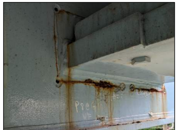
Photo 67: Reactivating surface corrosion on the west web at Girder 10
