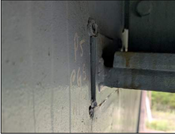
Photo 30: Retrofit in west web deflected up to 3/8" at Girder 5
