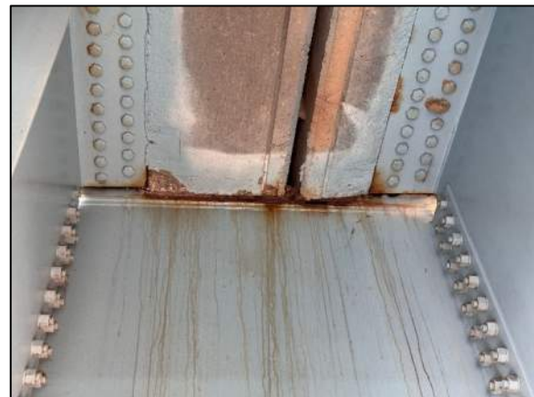
Photo 55: Layered corrosion on top flange and rust staining of the web plates due to leakage through the deck joint between Girders 5 and 6
