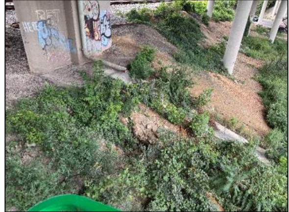
Photo 16: Erosion at the base of the north column
