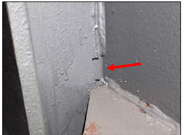
Photo 25: 1-1/2" discontinuity in weld between west web and a transverse stiffener between Girders 7 and 8
