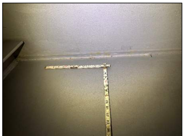
Photo 20: 33" long fillet weld between the top flange and east web between Girders 1 and 2
