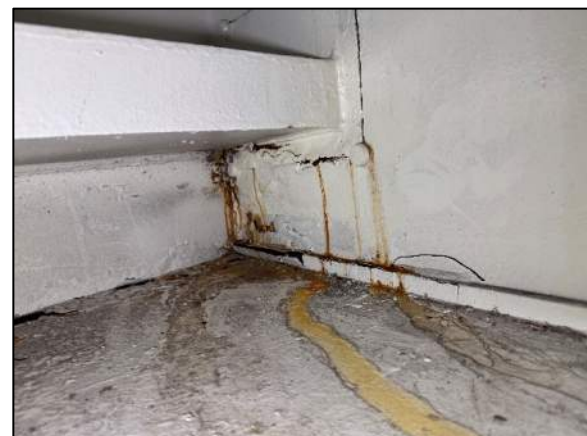
Photo 61: Bubbling paint and rust staining resulting from leakage through the web retrofit at Girder 10
