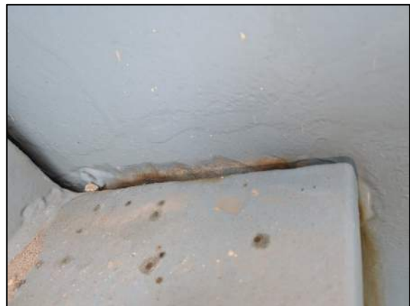
Photo 29: Reactivating corrosion at previously painted over section loss on east web at Girder 1.
