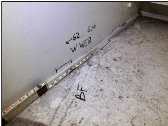
Photo 63: Random fillet welds between bottom flange and west web between Girders 1 and 2
