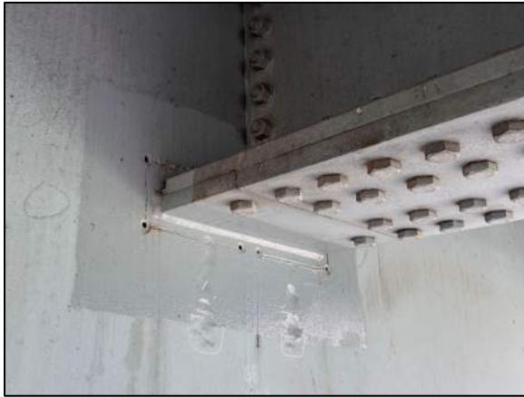
Photo 44: Heavy gouging on west web plate below Girder 8 from girder knee brace removal
