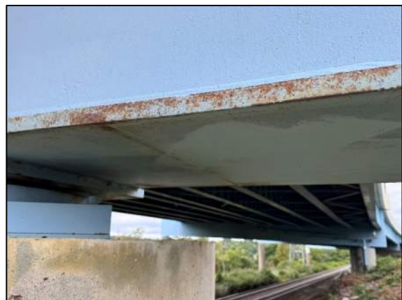
Photo 56: Surface corrosion along bottom flange
