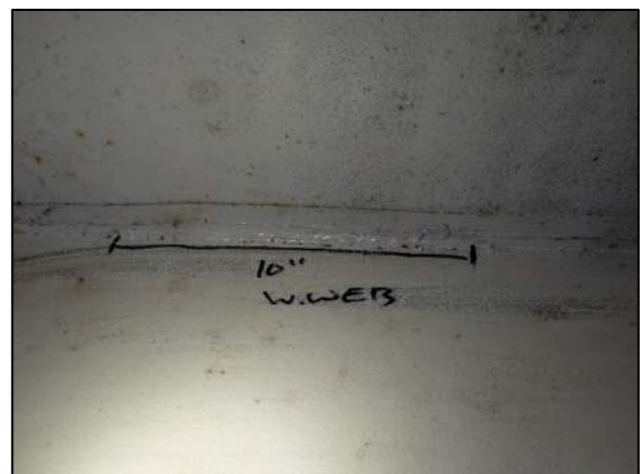
Photo 37: 10" fillet weld between the east web and top flange backer bar south of Girder 2
