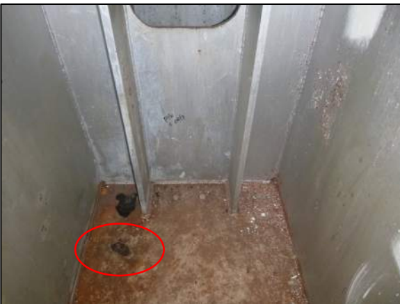
Photo 27: Feces encountered at east end above east bearing.
