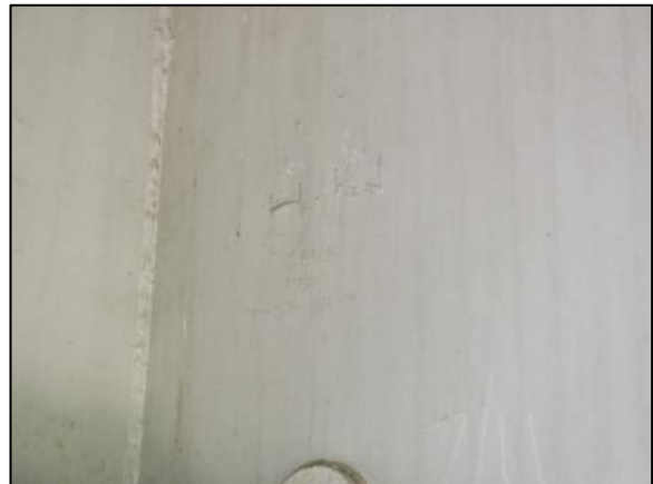
Photo 51: Tack welds on the south web of Pier Cap 20, east of Girder 3 above the girder flange
