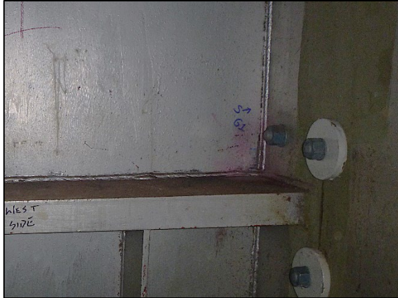
Photo 44: General location view of removed slag on Girder 1
