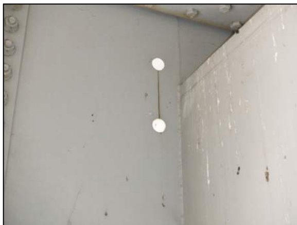
Photo 49: Numerous overcuts up to 1/8" on the Girder retrofits
