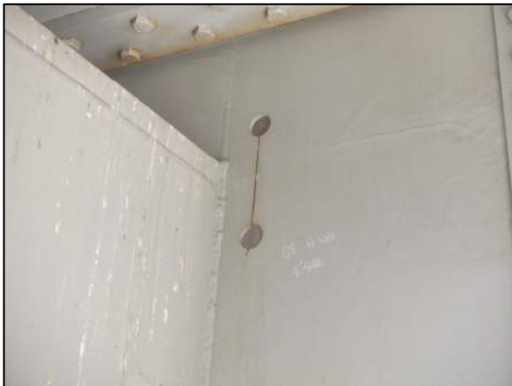
Photo 48: Sawcut retrofit extending 9/16" past stress relief hole on Girder 5 at the north web
