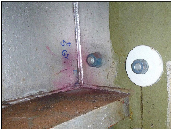
Photo 45: General location view of removed slag on Girder 1 (Closeup)
