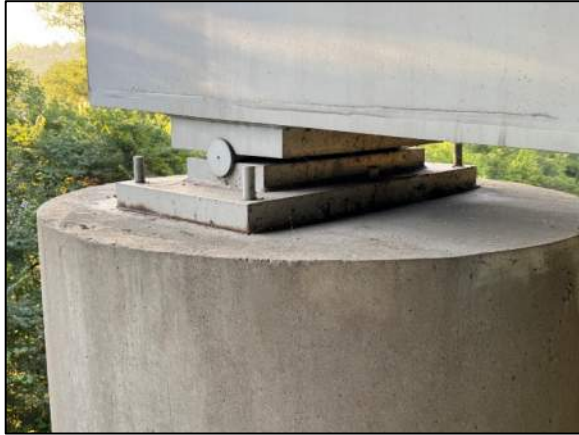
Photo 14: Typical Peeling Paint and surface corrosion at the east bearing of Pier Cap 5
