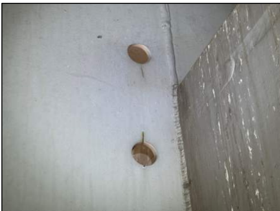
Photo 32: Stress relief holes in the web of Girder 4 at the north web of Pier Cap 16 not connected
