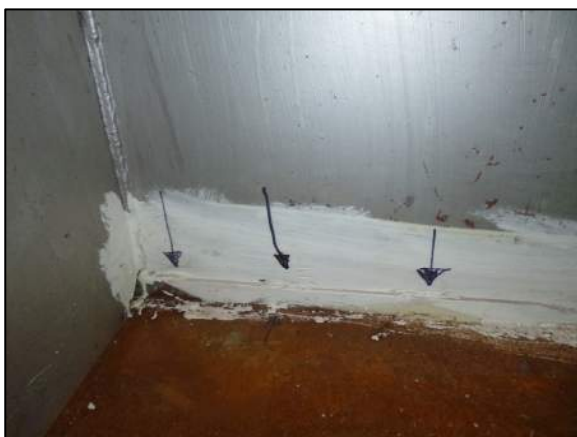
Photo 21: Typical partially removed tack welds on the bottom flange backer bar of Pier Cap 16
