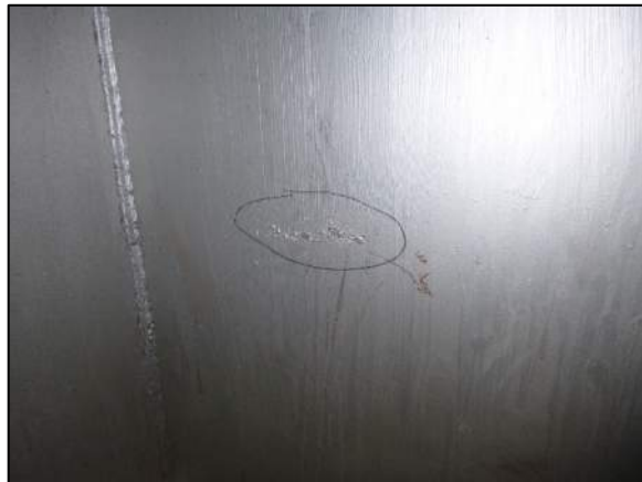
Photo 42: 4-1/2" of weld material on the south web of Pier Cap 20, east of the west bearing.
