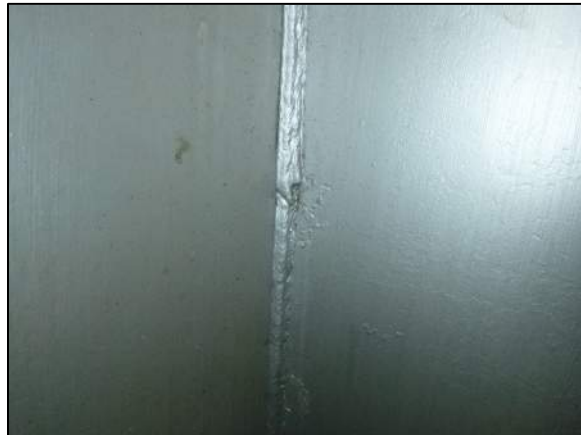
Photo 43: Sloppy welds at the diaphragms of Pier Cap 20
