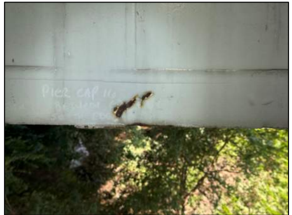
Photo 34: 4" tack weld between Girders 3 and 4 on the south face of the Pier Cap 16 bottom flange
