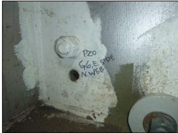
Photo 41: Unfilled stress relief hole above girder bottom flange east of Girder 6 at the north web
