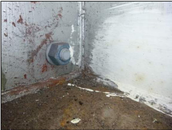
Photo 26: Typical triaxial weld above girder tie plate
