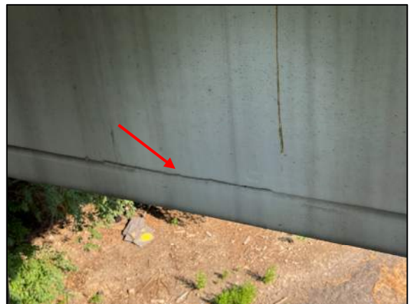
Photo 35: 18" overlapping weld under Girder 5 between the south web and bottom flange of Pier Cap 16
