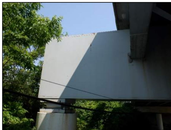
Photo 46: Bubbling paint and corrosion on the east face of Girder 7 extending onto the north web
