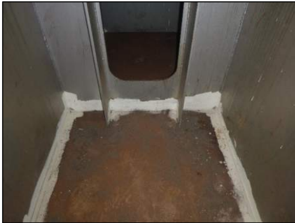
Photo 38: Typical light corrosion on the bottom flange of Pier Cap 20
