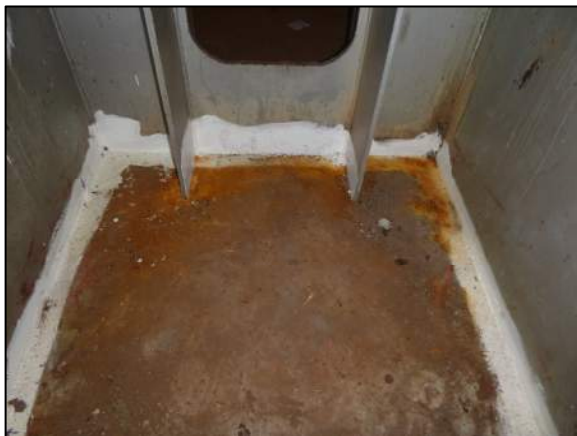
Photo 20: Typical corrosion and blasting media on the bottom of Pier Cap 16
