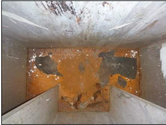
Photo 19: Corrosion on the bottom flange of Pier Cap 16
