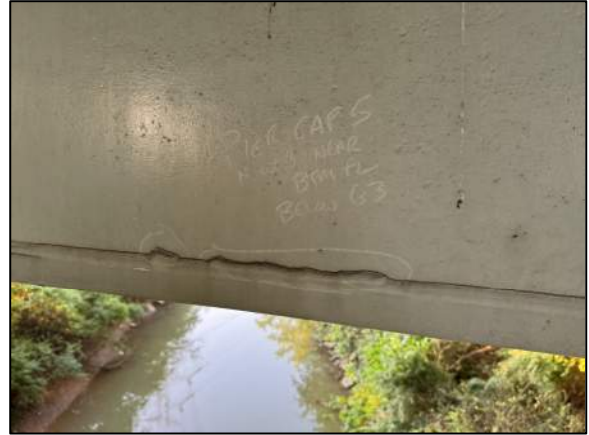
Photo 11: Fillet welds at groove weld between north web and bottom flange of Pier Cap 5, between Girder 2 and 3
