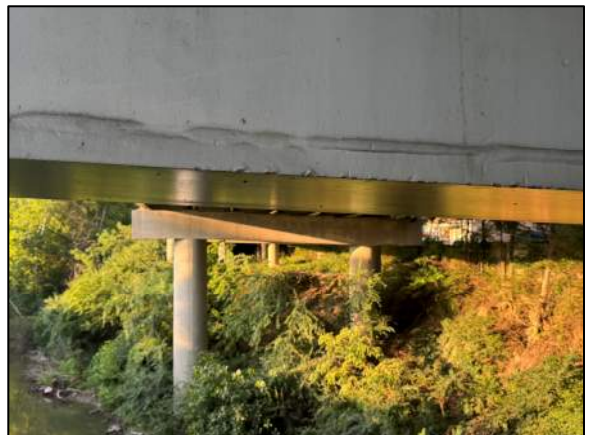
Photo 13: Gouges from construction on the north face of the bottom flange of Pier Cap 5 at Girder 2
