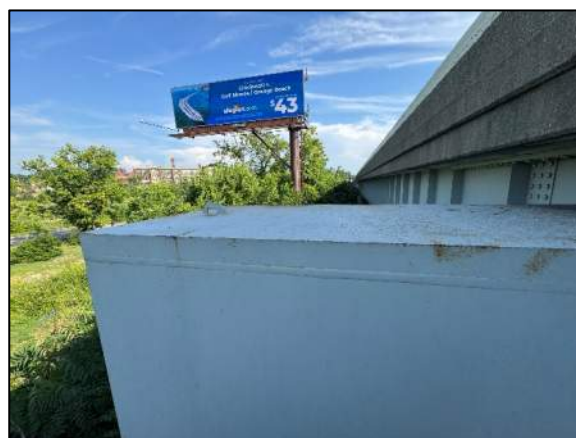
Photo 28: Typical freckling corrosion on the top flange at the west end of Pier Cap 16
