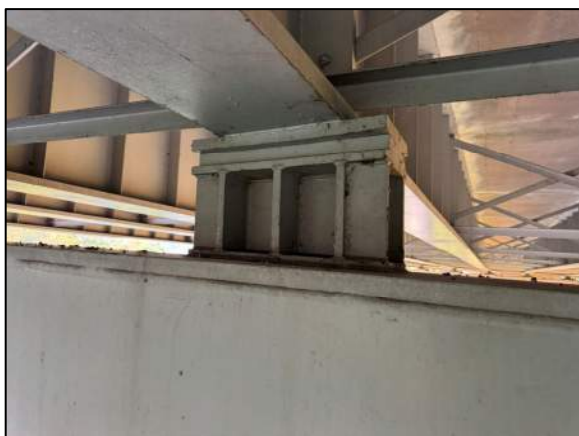
Photo 16: Surface Corrosion of the girder bearings at Pier Cap 5
