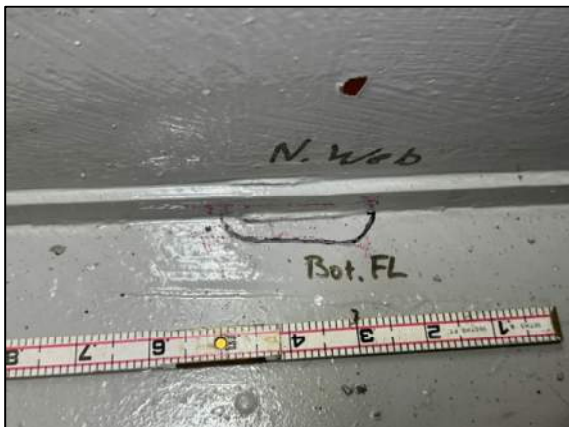
Photo 6: Typical 3" tack weld between the bottom flange and north web of Pier Cap 5, east of Girder 3
