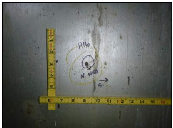
Photo 23: Random spot weld on the north web of Pier Cap 16, west of Girder 1
