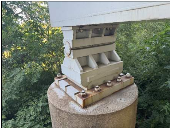
Photo 30: Surface corrosion on west bearing of Pier Cap 16
