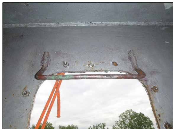
Photo 37: Two of the four missing nuts at the east access hatch of Pier Cap 20
