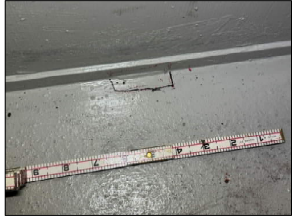
Photo 7: 2-1/4" tack weld between the bottom flange and north web of Pier Cap 5, west of Girder 3
