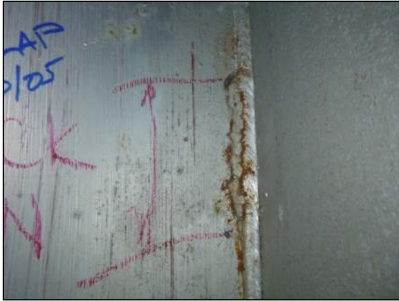
Photo 25: Typical excess weld bead material breaking off at overlapping welds
