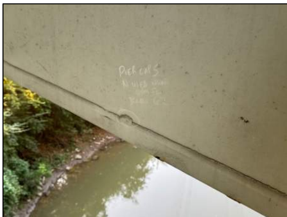
Photo 10: Typical overlapping weld beads on bottom flange of Pier Cap 5, south web below Girder 4
