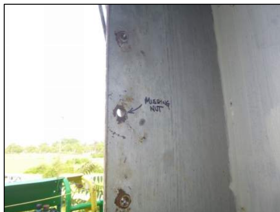
Photo 18: Missing nut for the west access hatch of Pier Cap 16
