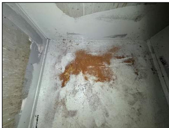
Photo 2: Surface corrosion on the bottom of the flange of Pier Cap 5 between Girders 3 and 4
