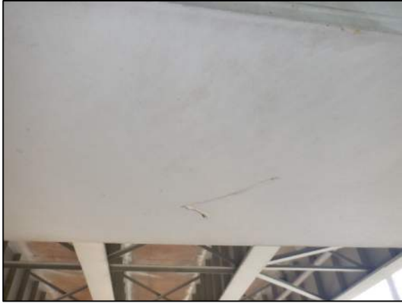
Photo 47: 14" Paint scrape due to impact on the bottom flange of Pier Cap 20 below Girders 5 and 6
