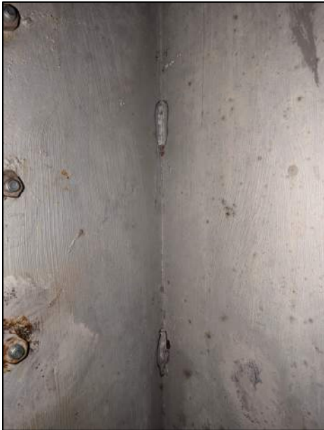
Photo 5: Tack welds ranging from 1.5" to 4" at the west end of the north end of Pier Cap 5
