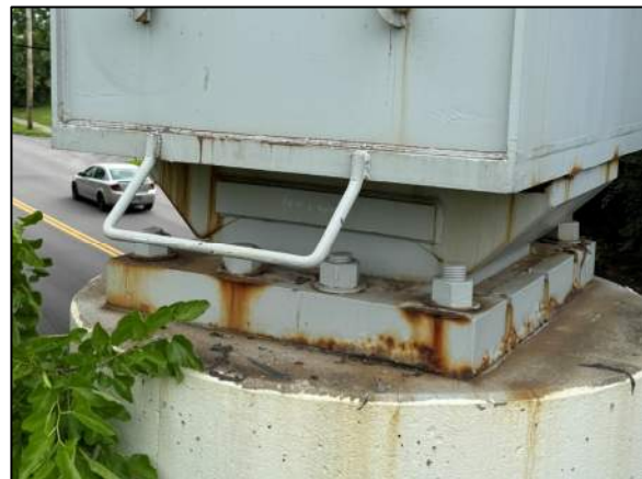
Photo 52: East Bearing cap Pier Cap 20 displaying peeling paint
