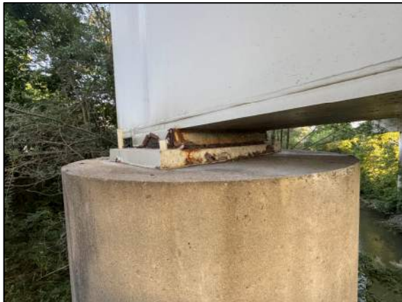
Photo 15: Typical Peeling Paint and surface corrosion at the west bearing of Pier Cap 5
