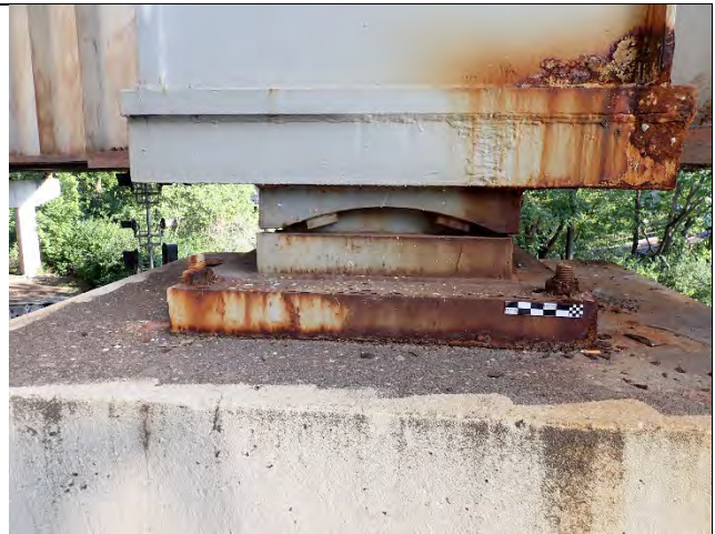
Photograph 17 –View of the South Bearing, Note Active Corrosion Continues, Heaviest On Masonry Plate. Looking North.
