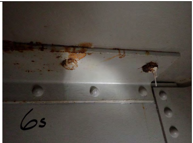
Photograph 4 – Example of Active Corrosion Through Bolted Clip Angle at Cap Top Flange
