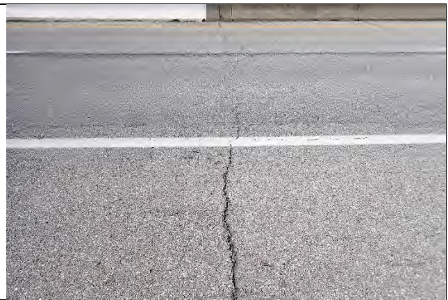
Photograph 36: Typical approach crack (eastbound shown), looking north.
