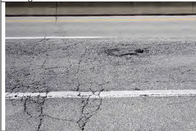
Photograph 37: Approach cracks and potholes (westbound shown), looking north.
