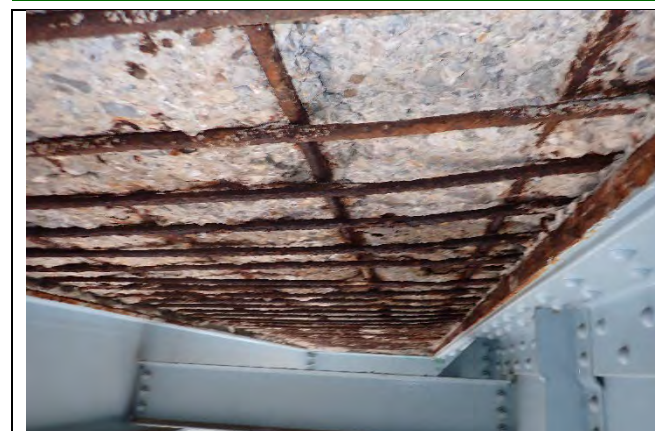
Photograph 5: Span 3 soffit near Girder 1 south side between Floor Beams 2 and 3, looking west. Note: all transverse reinforcing bars were not engaged with the soffit, and section loss was observed on each with 1 bar fully severed.
