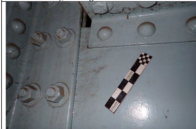
Photograph 13: Typical localized painted over pitting of 1/16 in. on the knee brace web plates at angle connections to the girders (Span Girder 1 at Forward Abutment shown), looking east.
