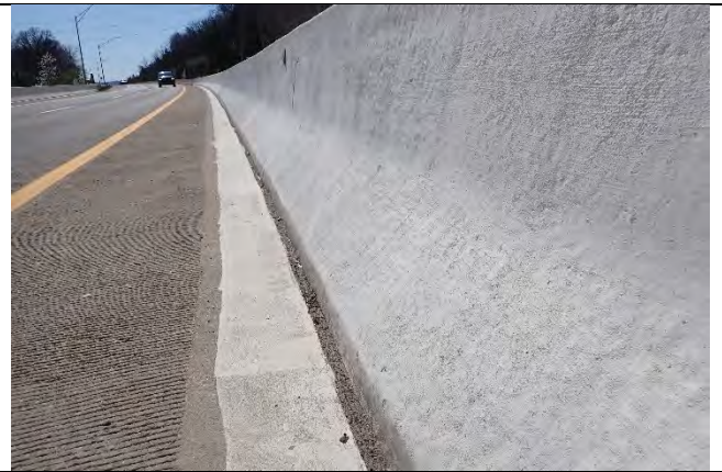
Photograph 44: View of joint along median for eastbound bridge, looking west. This is where the leakage between the bridges is coming through.
