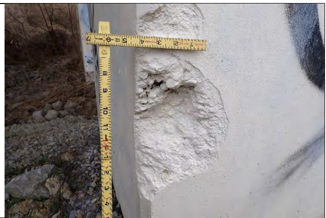
Photograph 24: Pier 1 Column 1 shallow spall, looking south.
