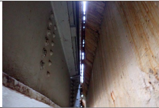
Photograph 28: Forward Abutment deck header spalling and joint failure, looking east.
