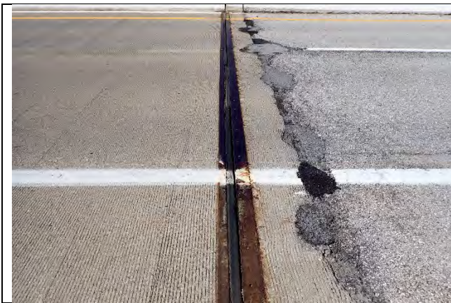
Photograph 35: Eastbound east joint with potholes, looking north.
