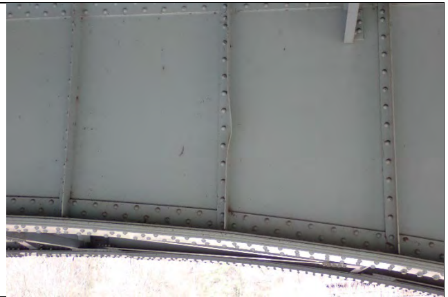
Photograph 16: Close up of vertical stiffener bent approximately 2.5 ft above the bottom flange (Span 2 Girder 2 south face), looking north.
