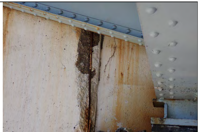
Photograph 40: Spall in Rear Abutment backwall, looking west.
