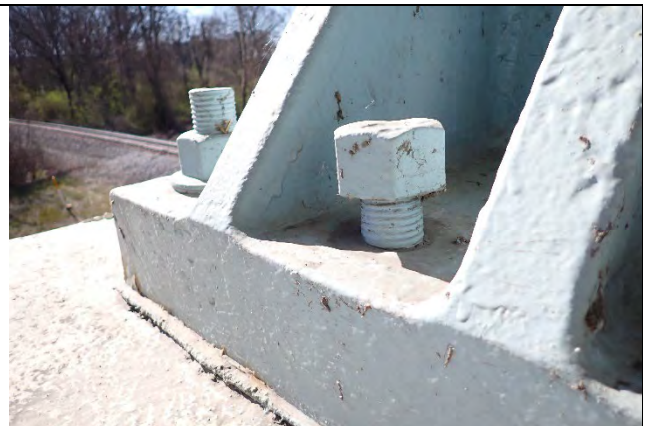
Photograph 22: Loose nut at the Girder 4 bearing at Pier 2, looking south.
