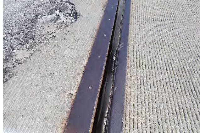
Photograph 30: Close up view of torn and fallen joint seal (Forward Abutment westbound right lane shown), looking south.
