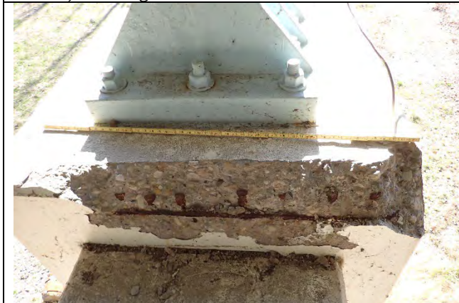
Photograph 25: Pier 2 Column 4 spall near the bearing seat, looking south.
