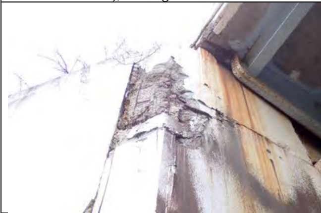
Photograph 45: Spalled area at top corner of southwest wingwall at the abutment with exposed rebars and wire mesh, looking northwest.
