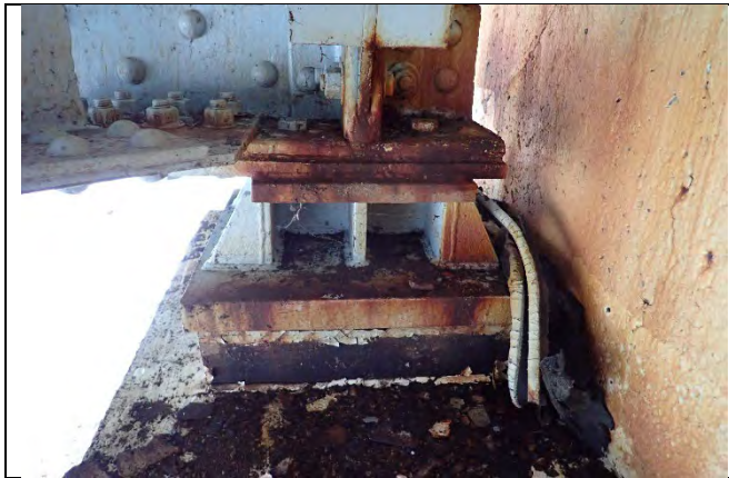
Photograph 20: Girder 2 Rear Abutment bearing with typical example of rust staining on beam and bearing, looking south.
