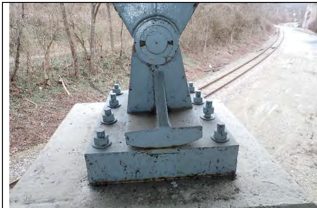
Photograph 21: Girder 1 bearing at Pier 1 with an improperly seated anchor nut, looking north.
