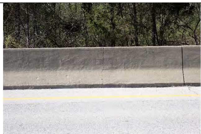
Photograph 42: West approach median parapet cracking, looking north.
