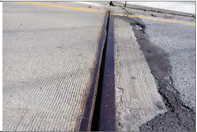
Photograph 29: Failed westbound left lane joint seal at the Rear Abutment, looking south.
