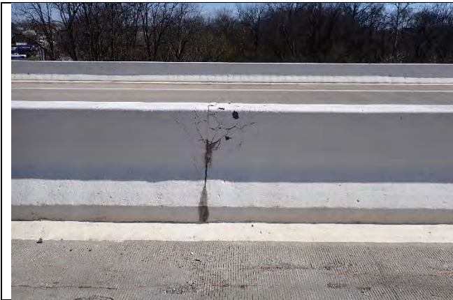
Photograph 43: General example of map/random cracking and deterioration of median (Span 1 westbound shown), looking south.
