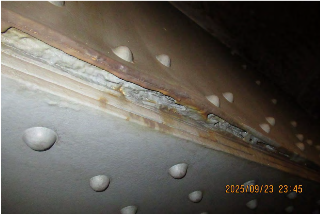
Photo 69 - Pack rust between box cap web and bottom flange at Pier 8A. Note: Pack rust has been painted over.
