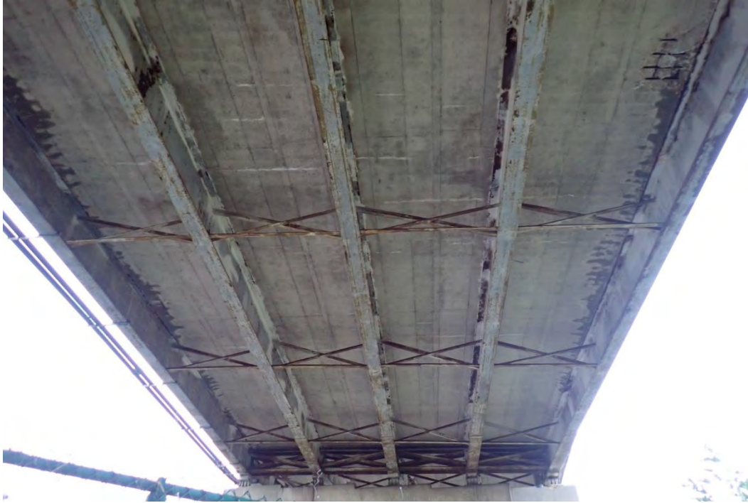
Photo 102 - Typical protective coating failure, with minor surface corrosion, and chalking from Pier 15A to Pier 28B. Photo of Span 27B, looking north.
