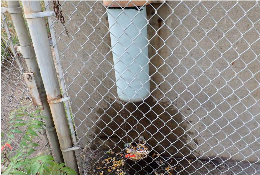
Photo 24 - Drain pipe impacted with debris and disconnected at base at Pier 6A, looking west.
