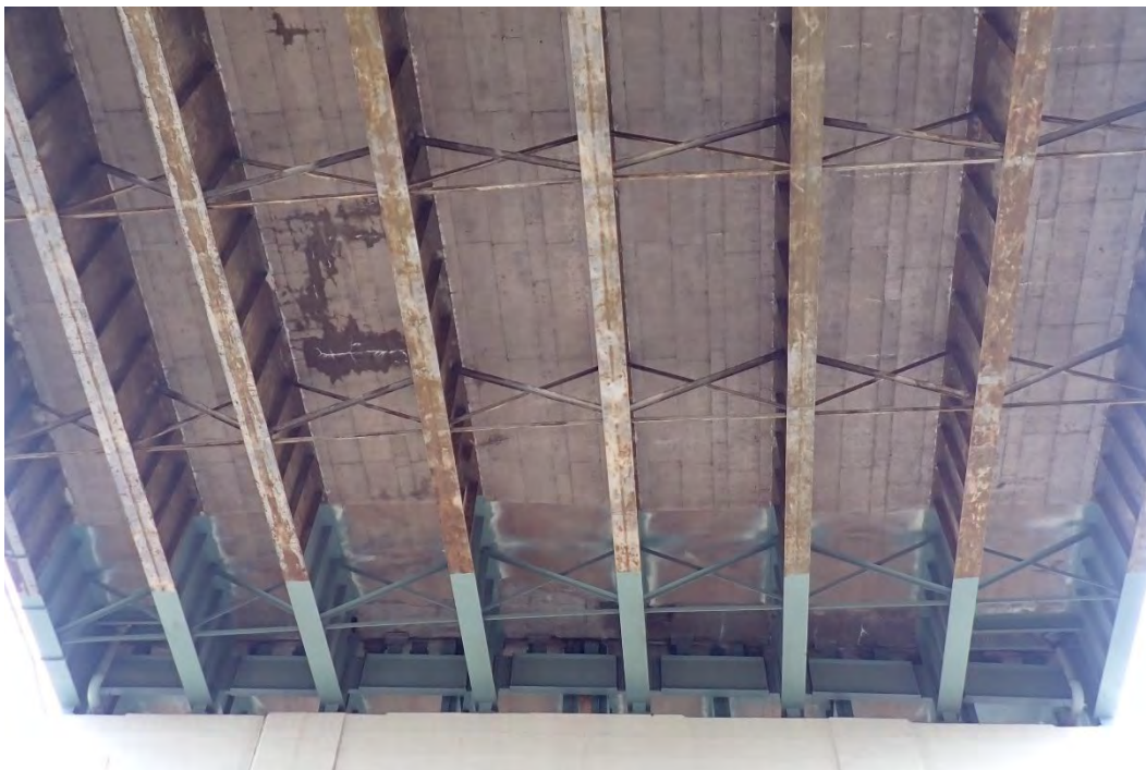
Photo 101 - Superstructure paint condition near deck joint at Pier 19A, looking north.
