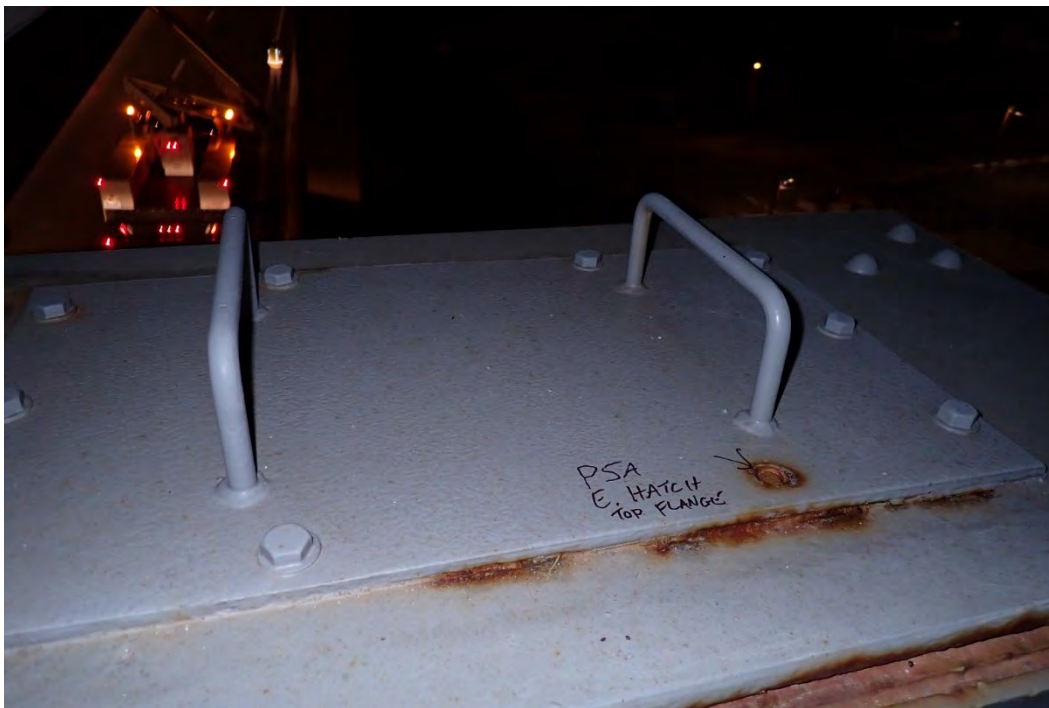
Photo 60 - Typical top hatch access to box cap interior, with missing bolt at Pier 5A, looking north.
