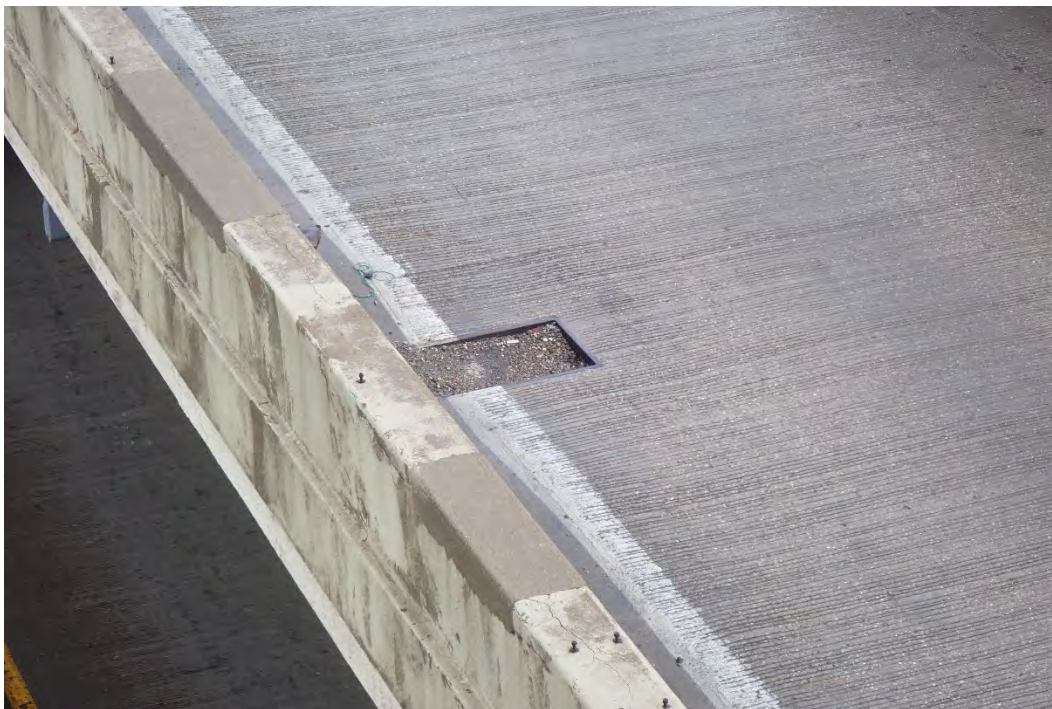
Photo 25 - Missing deck drain grate with debris accumulation at Span 2A, looking northeast.
