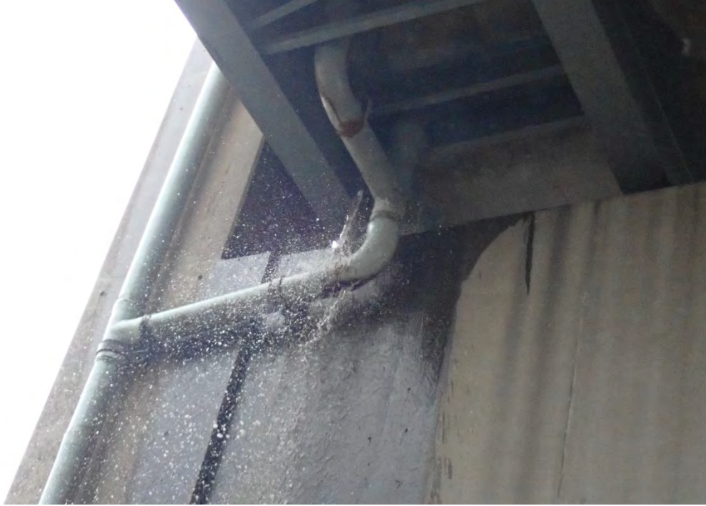
Photo 28 - Clogged and overflowing drainpipe at Pier 2A, looking south.
