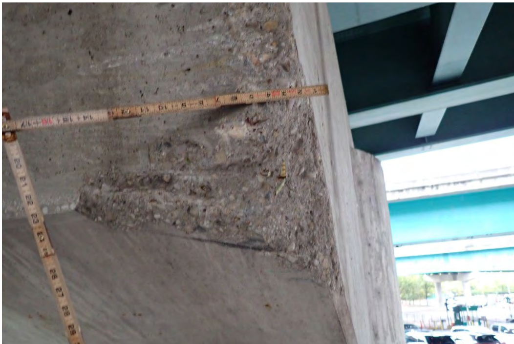
Photo 122 - 24" wide by 24" high by 4" deep corner spall with exposed reinforcement at Pier 2 (FWW).
