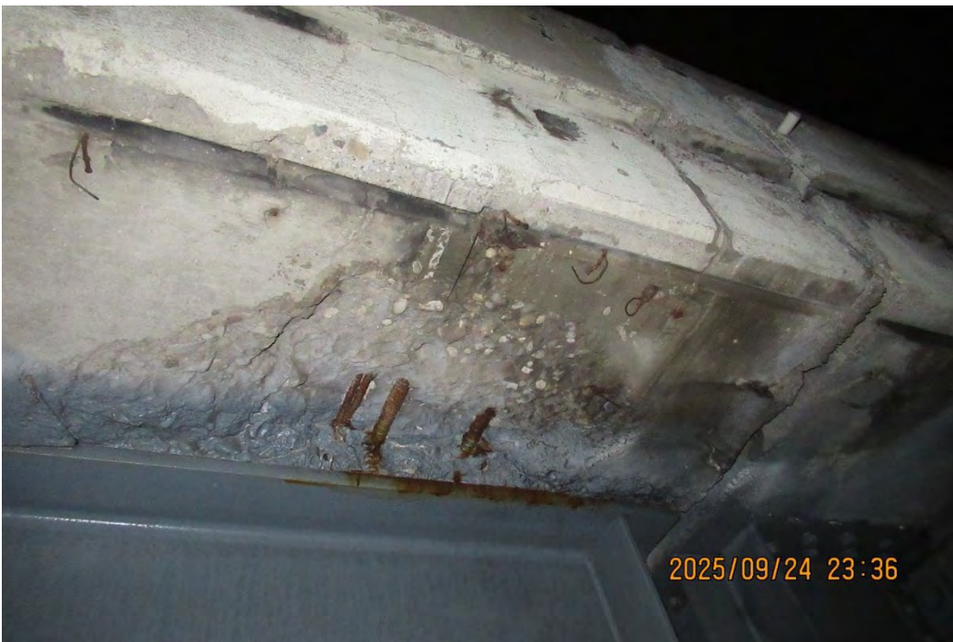
Photo 10 - 5' long by 20" wide by 5" deep spall with exposed rebar in the east overhang, both near midspan of Span 8A.
