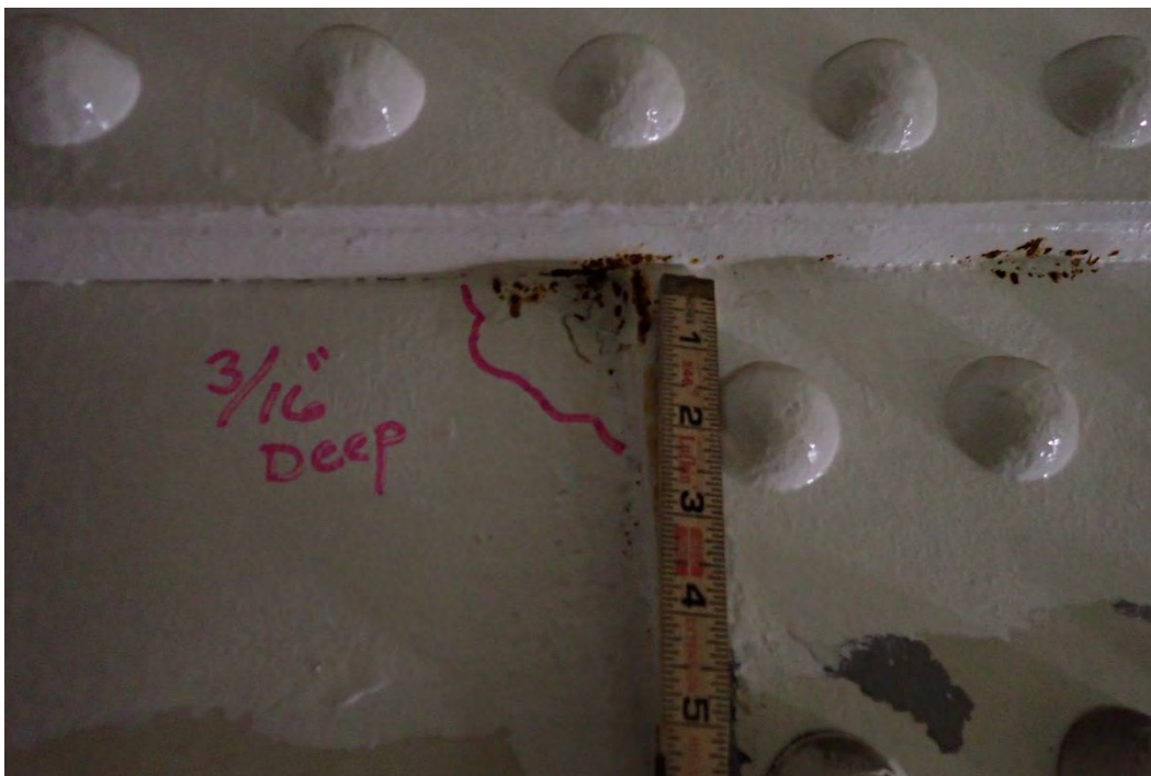
Photo 81 - 1" diameter area of up to 3/16" deep pitting on south web at splice plate.
