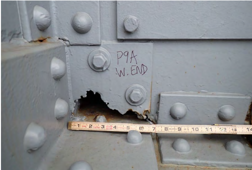
Photo 73 - 100% section loss of a bolted and welded keeper plate approximately 6.5" x 3" at the west end of Pier 9A's box cap, looking east.
