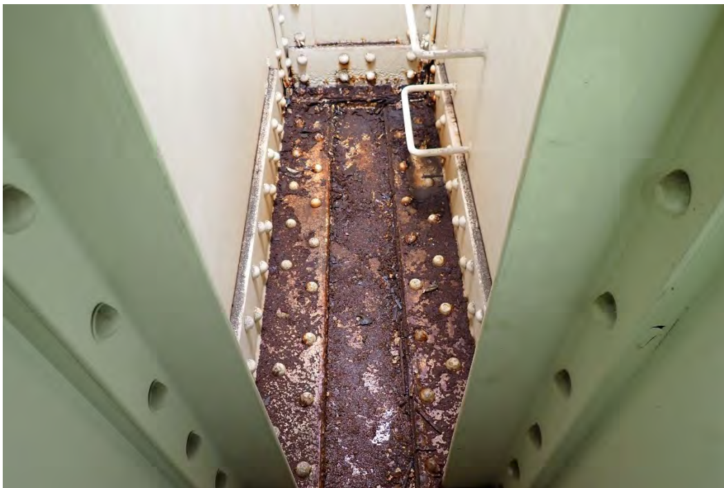
Photo 74 - Bottom surface of box cap covered by up to 1/2" of granular debris and dust that is rusting from moisture.
