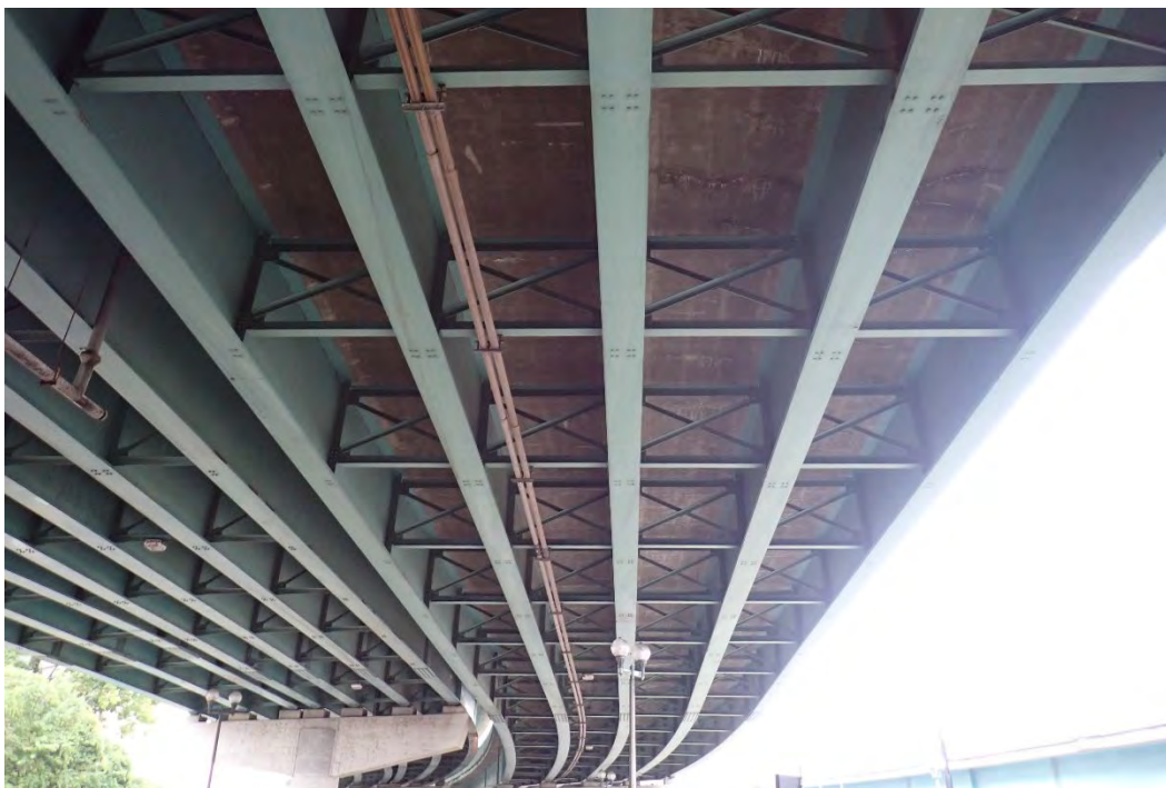
Photo 39 - Typical girder layout and condition at FWW Span 4, looking southeast.
