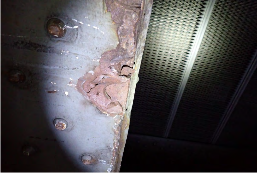
Photo 49 – Impact damage and corrosion with minor section loss, with missing rivet from bottom flange over center lanes on Pier 1A, looking northeast.
