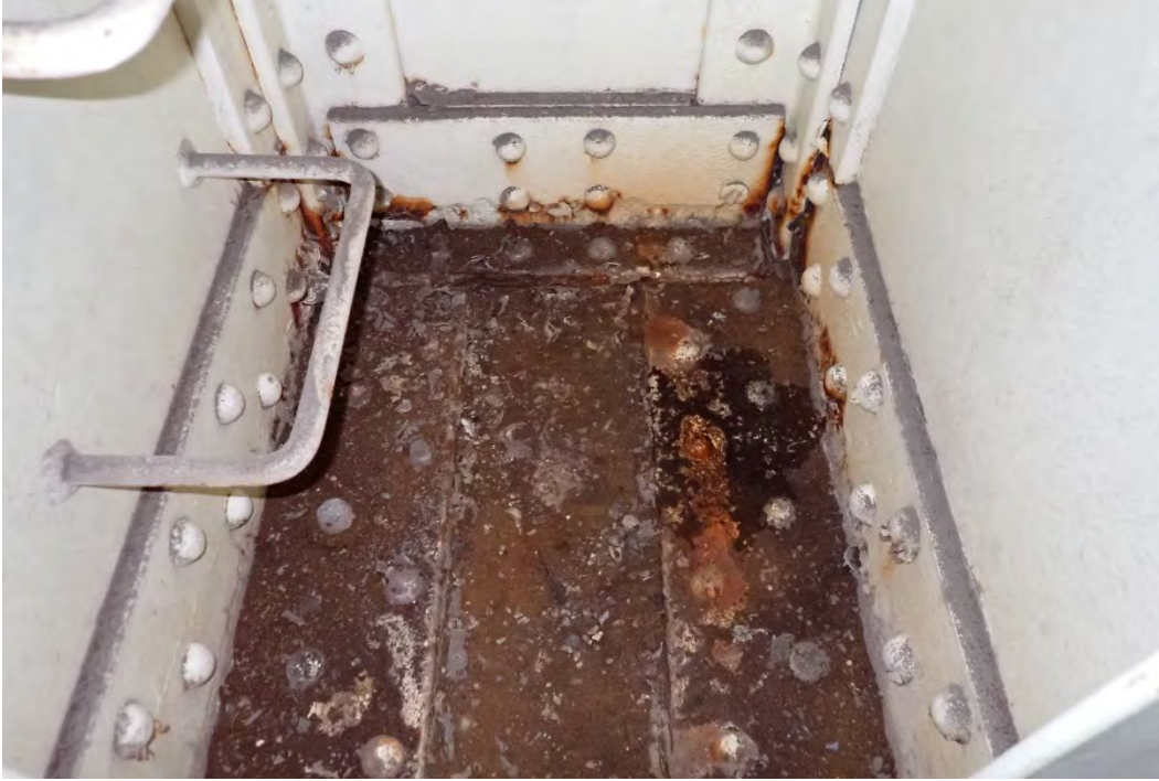
Photo 52 - Typical dry box cap interior with light surface corrosion at Pier 2A, looking east.
