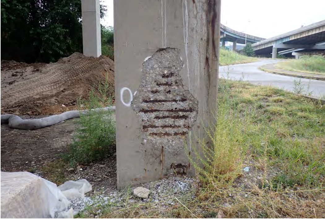
Photo 119 - Large spall with rebar on east column of Pier 23B, looking northwest.
