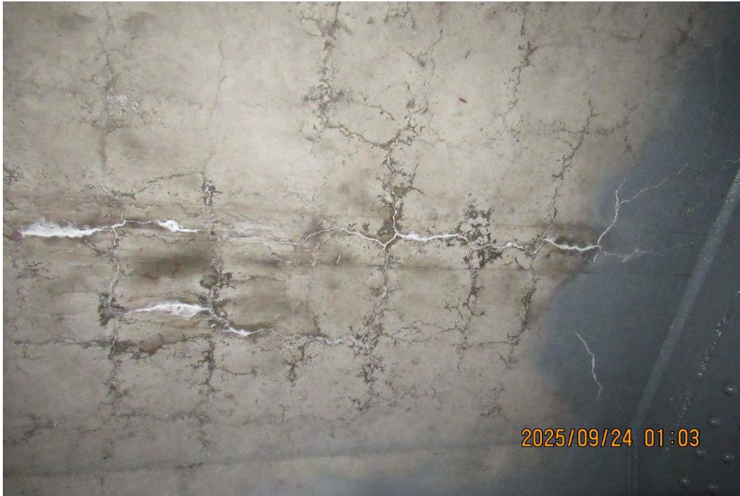
Photo 3 – Typical transverse cracking with efflorescence throughout girder bay sat Span 11A Bay 4, looking west
