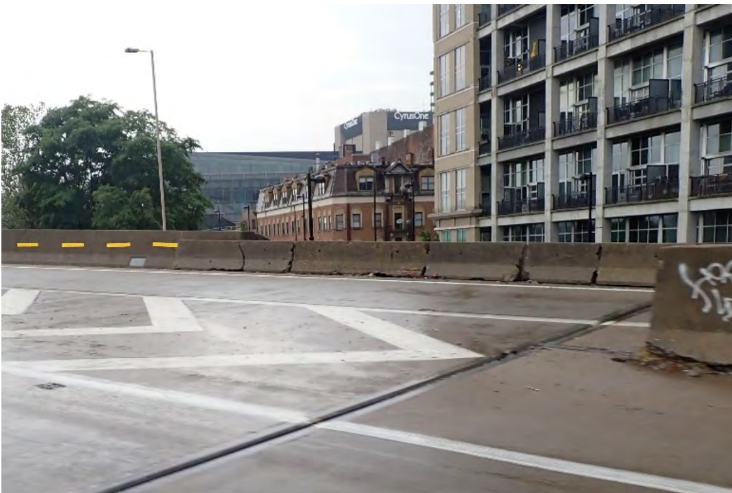
Photo 19 - Wide vertical cracks in concrete railing on west railing or Span 5.
