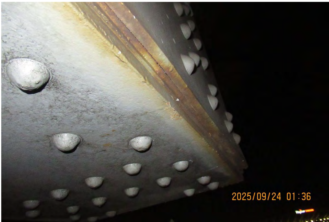
Photo 82 - 3/8" thick pack rust between both web plates and bottom flange angles that has been previously caulked and painted.
