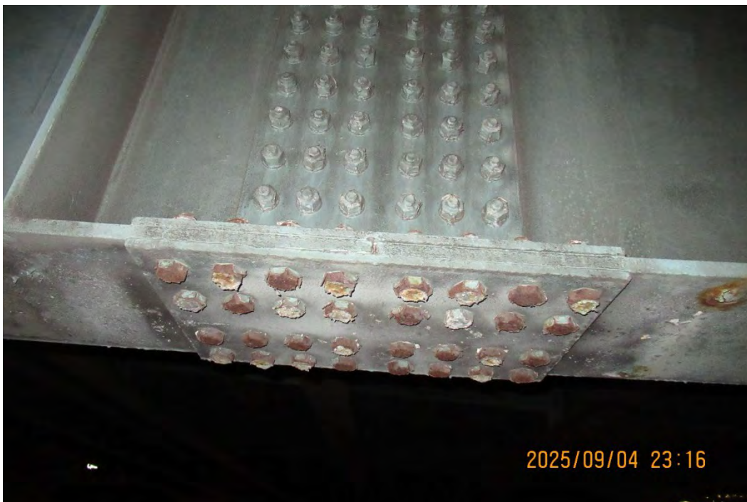
Photo 88 - Typical surface corrosion at pier cap bolted splice connection on Pier 29B.
