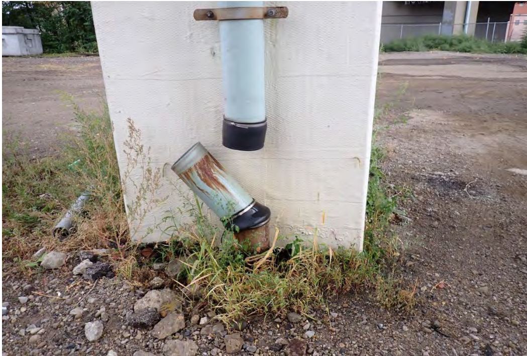
Photo 26 - Typical disconnected drainpipe at pier column base at Pier 19A, looking south.
