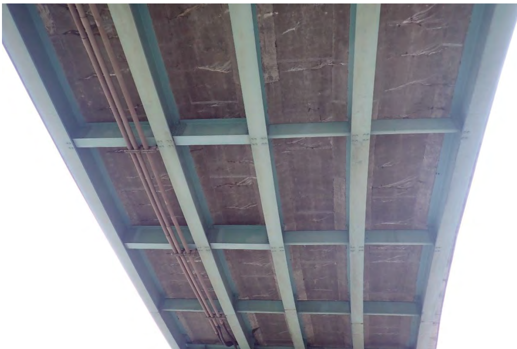
Photo 6 - Typical transverse cracking with efflorescence on deck underside at Span 29B, looking northeast.
