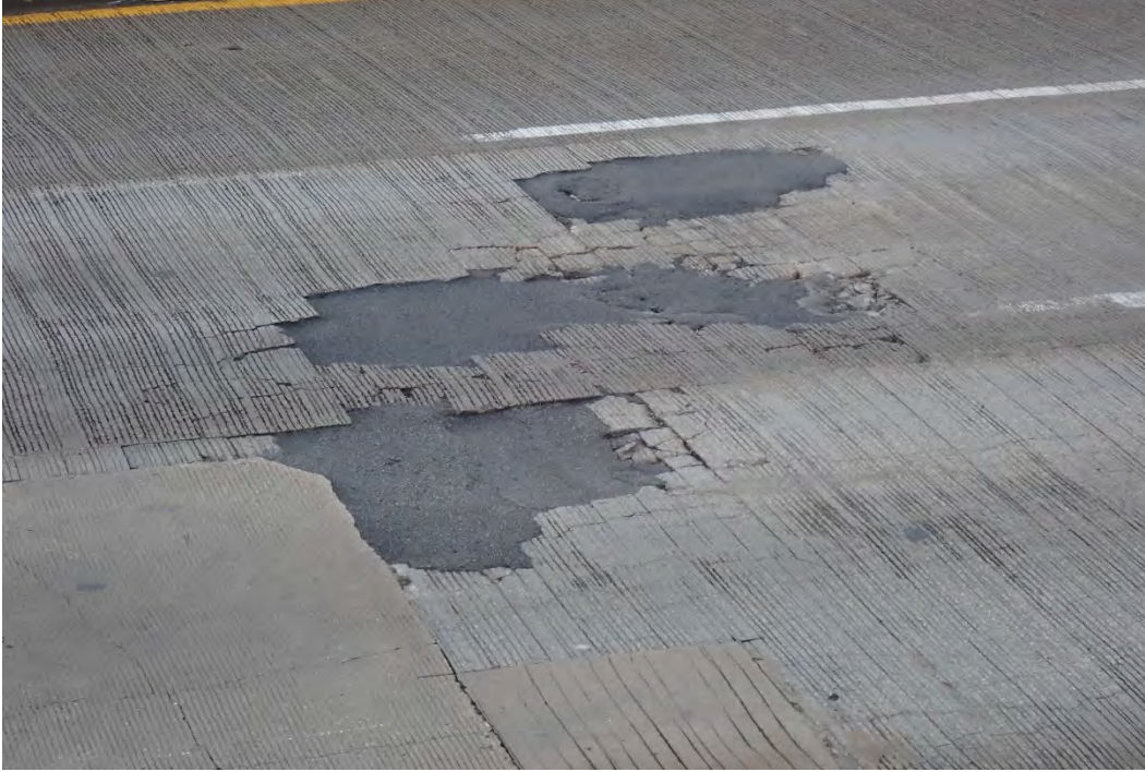
Photo 14 - Typical asphalt patching of pothole in deck at Span 8A, looking east.
