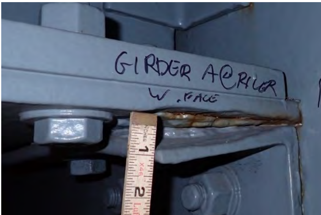
Photo 33 - 1" of pack rust between girder and bottom flange angle at River Pier Girder A, looking southwest.
