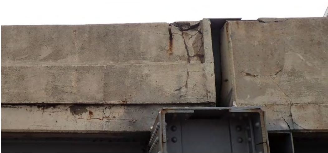
Photo 22 - Spall with exposed reinforcement, surrounded by delaminated concrete, at the River Pier, looking east.
