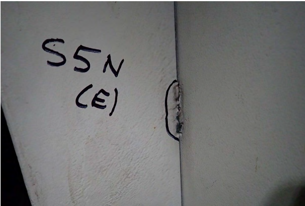
Photo 50 - Typical tack weld between box cap web and interior stiffeners at Pier 1A, looking west.
