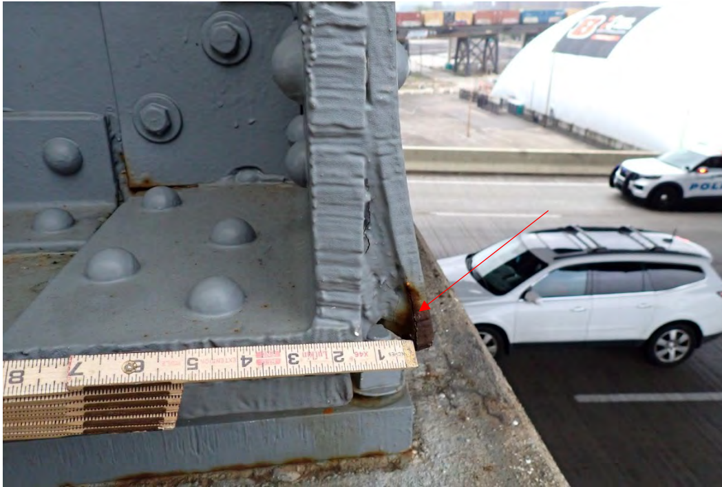
Photo 71 - 1/8" pack rust at the west end of Pier 9A's box cap, looking east.
