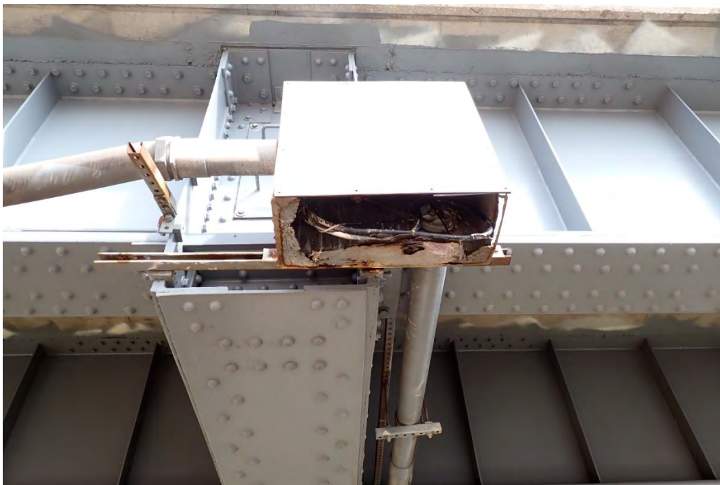
Photo 125 - Utility box with bottom 100% corroded on Pier 13A, looking east.
