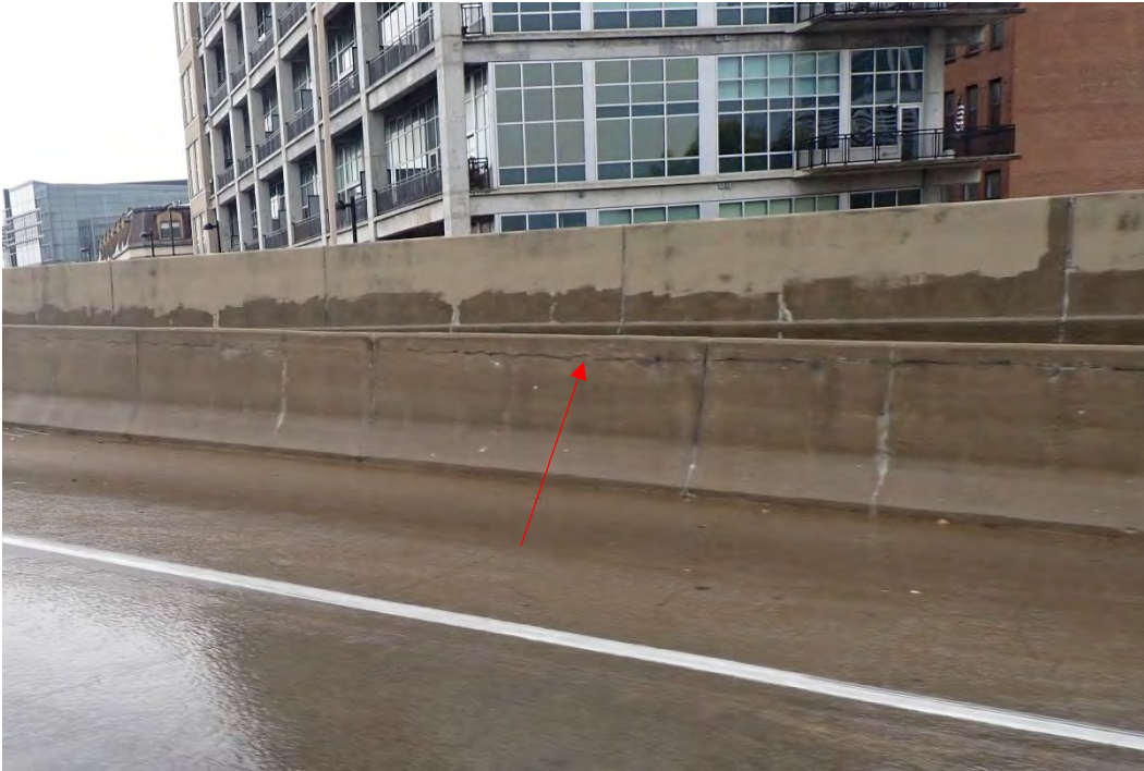
Photo 18 - Typical longitudinal cracking along top of concrete bridge railing.
