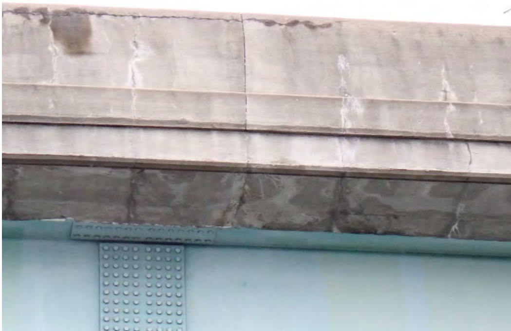
Photo 17 - Typical concrete bridge railing with vertical hairline cracking and efflorescence at Span 3, looking northeast.
