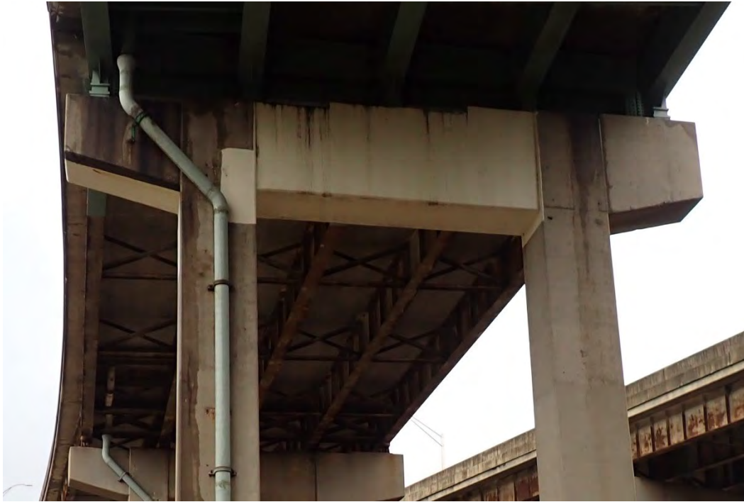
Photo 123 - Failing/peeling protective coating at Pier 23B, looking south.
