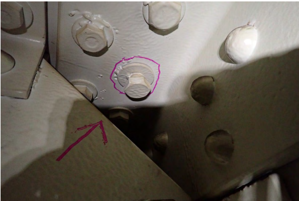
Photo 46 - Not fully seated bolt at the south top flange angle of Girder E, looking east.
