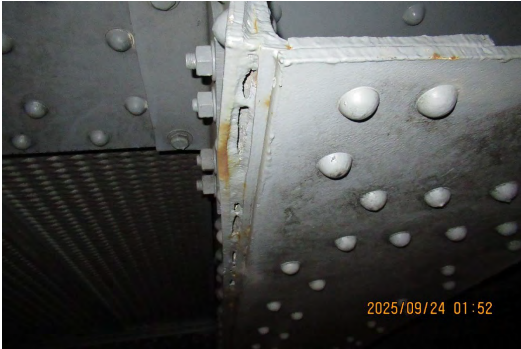
Photo 84 - Painted over pack rust up to 1" at the south web of Pier 13A's box cap, looking west.
