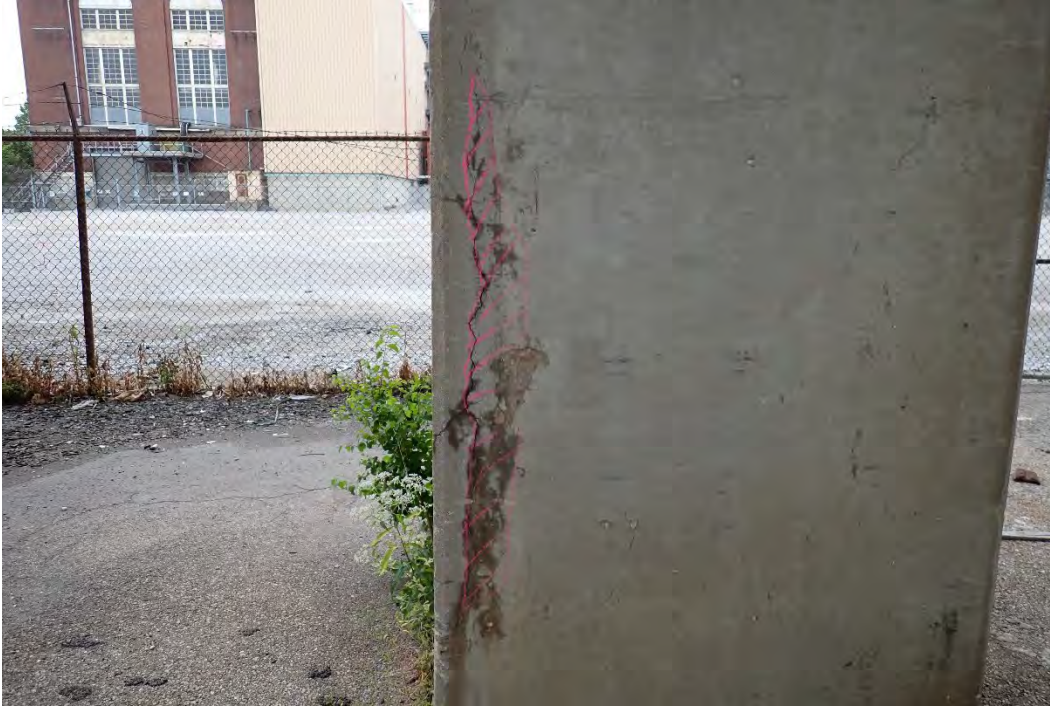
Photo 115 - Minor spalling and delamination on west column of Pier 1A, looking west.
