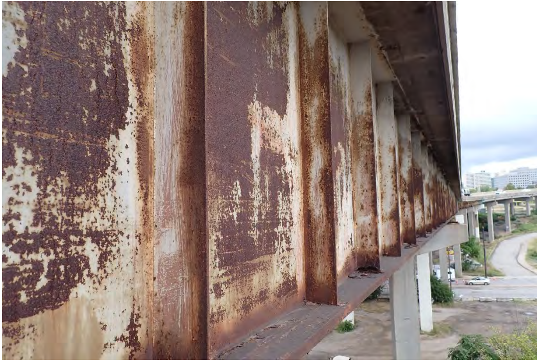
Photo 36 - Typical surface corrosion and pack rust in webs and bottom flange of girders at Span 18A east facia girder looking north.
