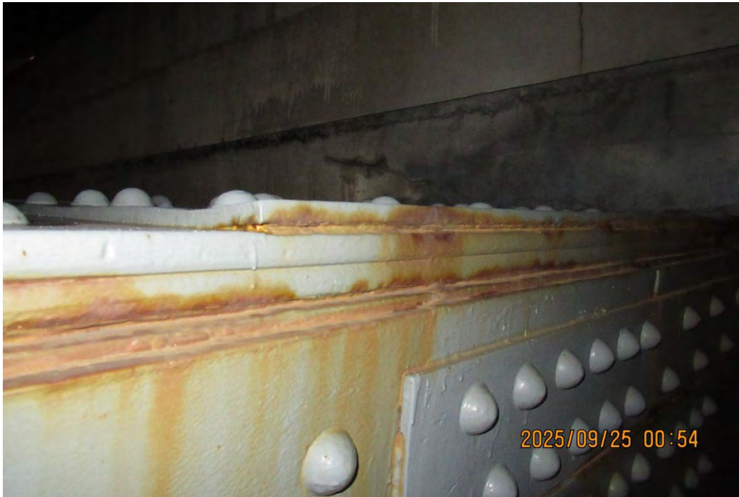
Photo 76 - 1/4" of pack rust on box cap cover plates of Pier 10A, looking south.
