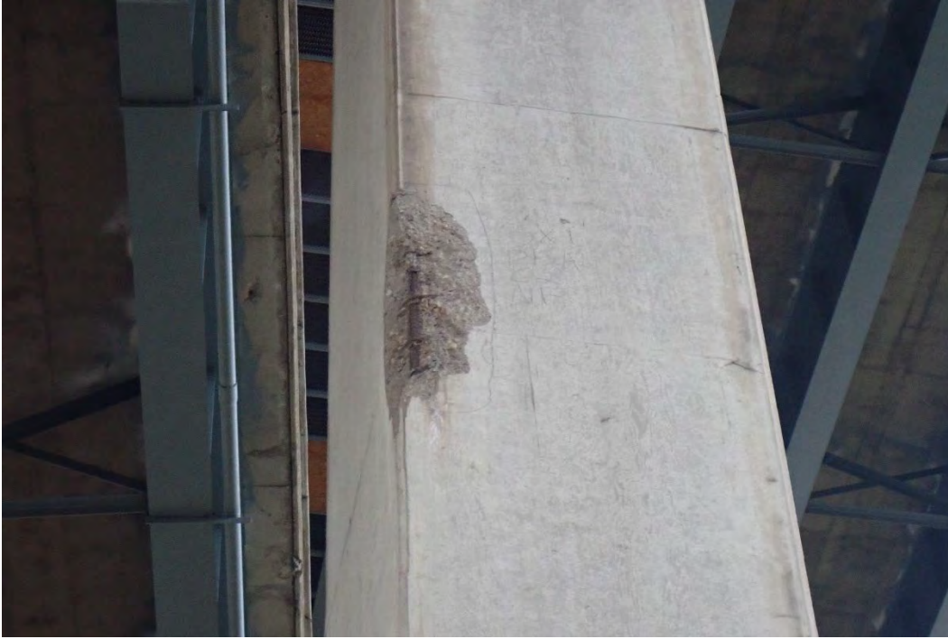
Photo 117 - Large corner spall with rebar on the east column of Pier 13A, looking south.
