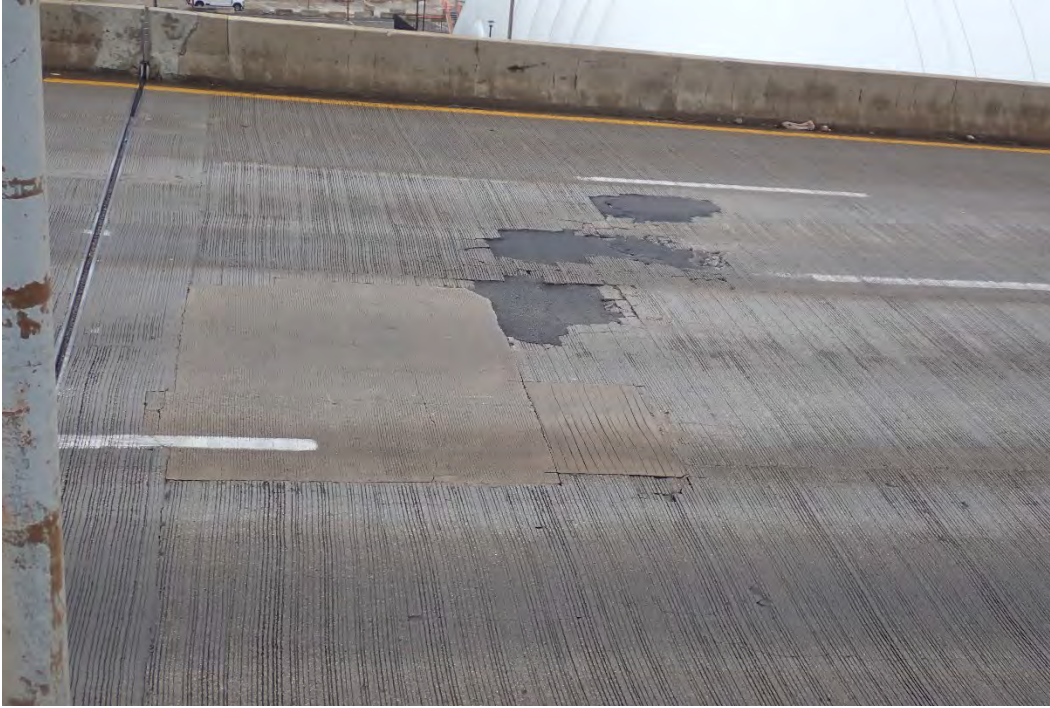
Photo 7 - Pothole in top of deck with temporary asphalt fill/patch at Span 8A, looking east. Note: previous deck repair.
