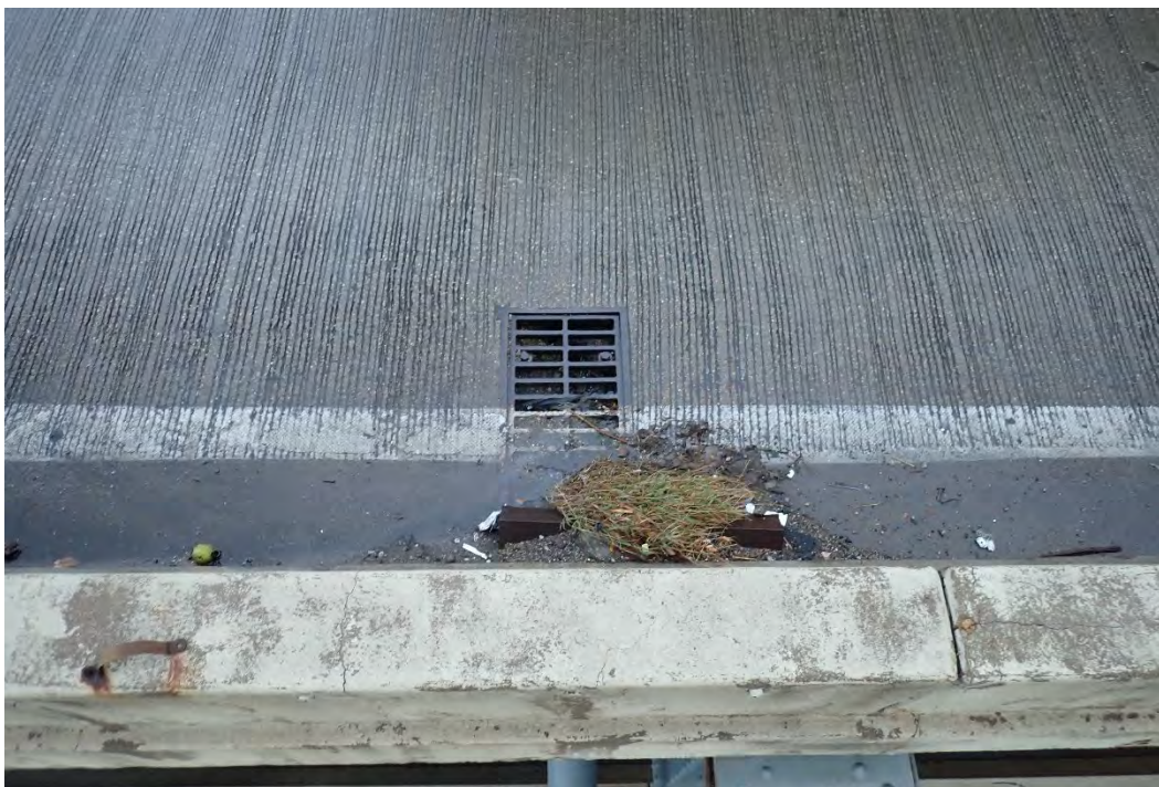
Photo 23 - Debris impacted deck drain with vegetation growth at pier 6A, looking east.
