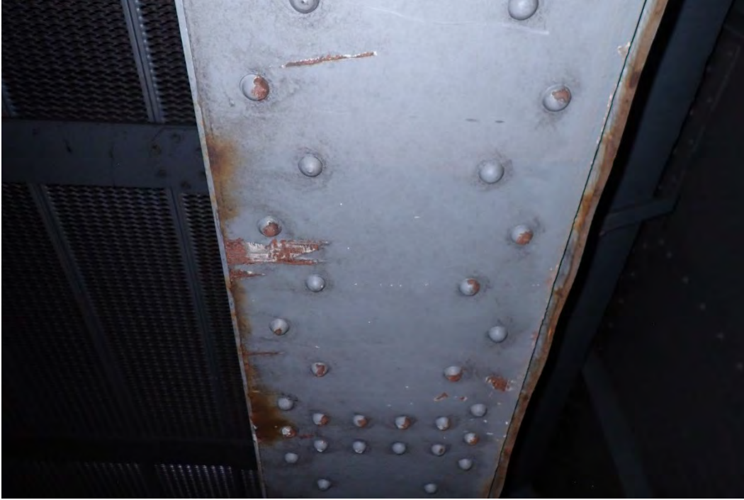
Photo 45 - Impact scrapes to bottom flange and rivets removed protective coating on River Pier, looking east.
