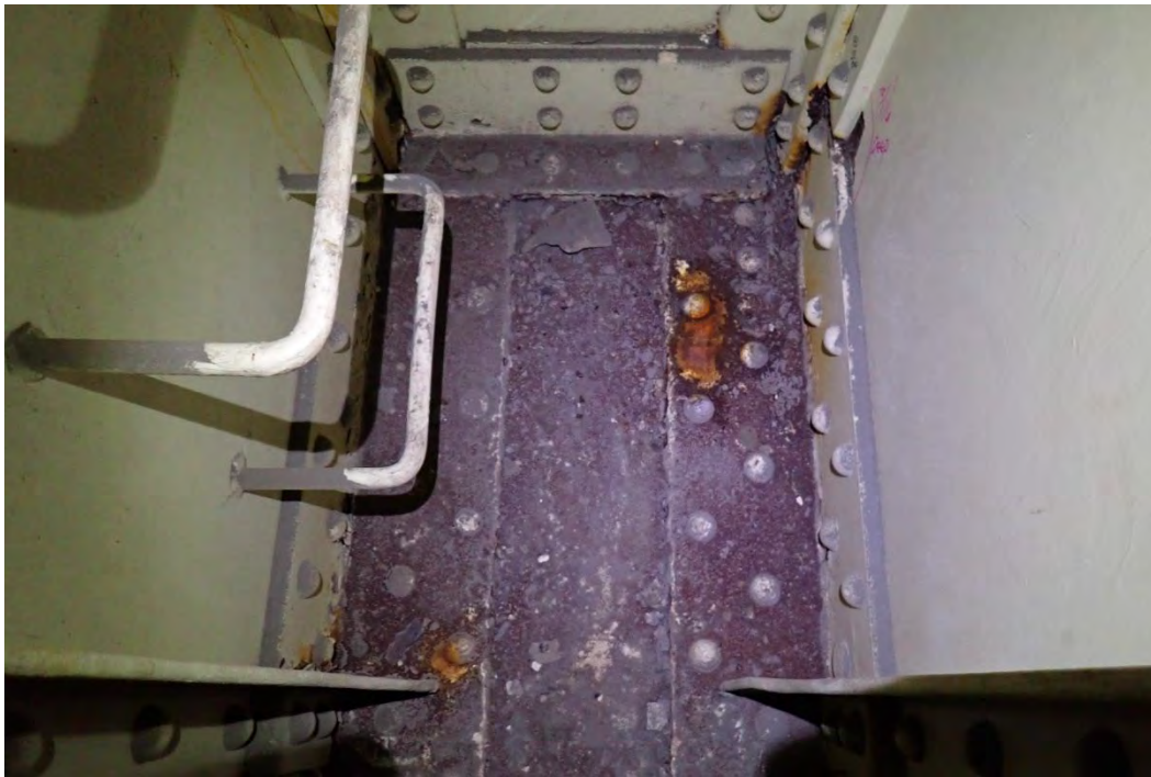
Photo 53 - Typical interior corrosion with pitting of bottom flange in box cap at Pier 3A, looking east.
