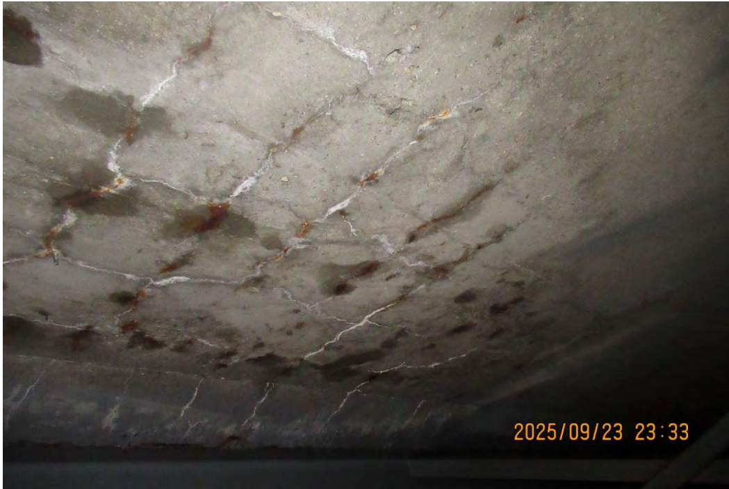
Photo 5 - Hairline transverse and map cracking with efflorescence at the underside of Deck in Span 8A.
