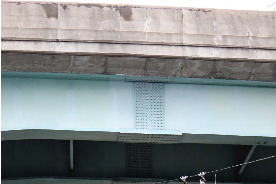
Photo 9 - Typical deck overhang at Span 3, looking north. Note: minor transverse cracking along with efflorescence.
