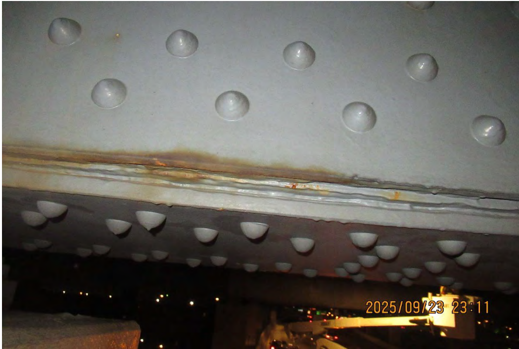
Photo 67 - 1/2" of pack rust between box cap web and bottom flange at Pier 7A. Note: Pack rust has been painted over.
