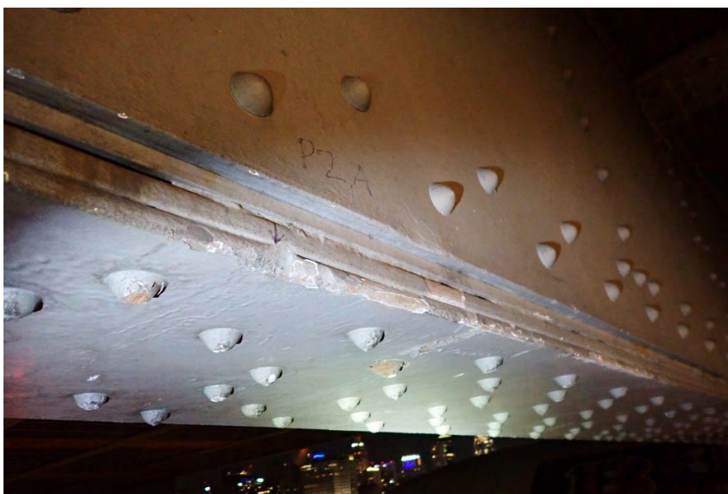
Photo 51 - Minor impact damage and scrapes along bottom flange of box cap at Pier 2A, looking northeast.
