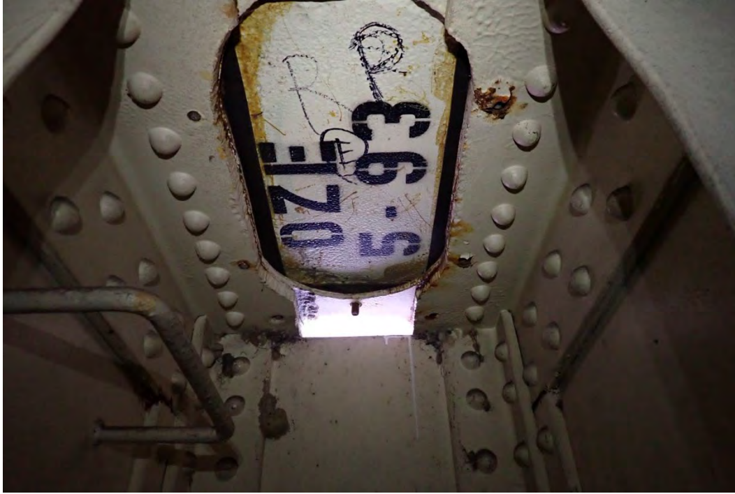
Photo 47 - Minor areas of freckled rust around top hatch at east end of box cap at River Pier, looking east.
