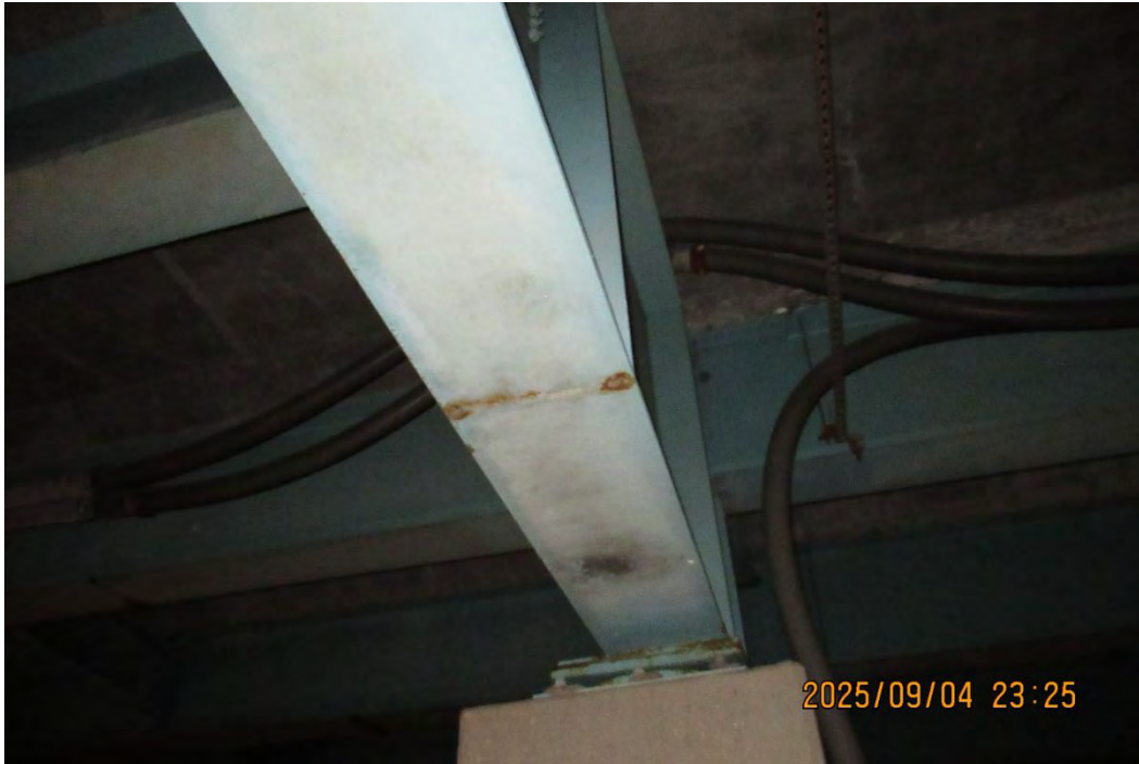
Photo 87 - Surface corrosion of the bottom flange at stiffener plate weld on north end of pier cap, at Pier 29B
