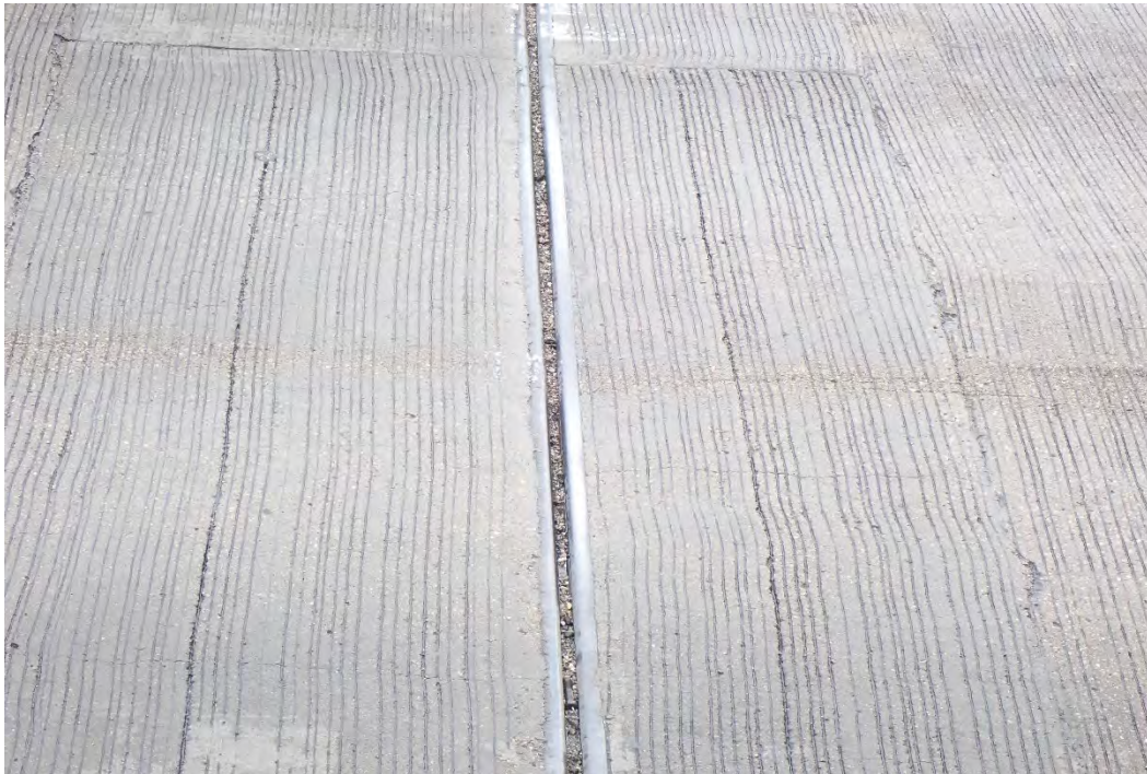
Photo 15 - Typical debris accumulation in expansion joint at Pier 4A, looking east.
