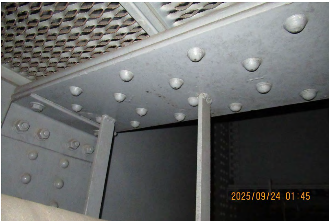
Photo 37 - Drain pipe hangers welded to the bottom flange of Girder E at Pier 12A, looking southeast.
