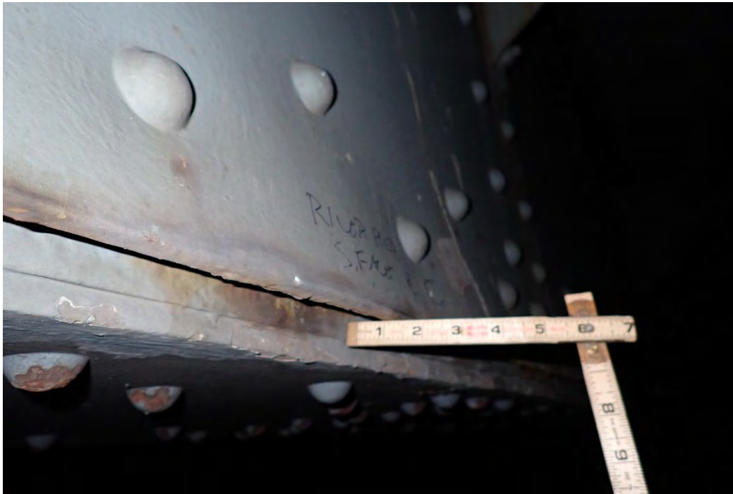
Photo 44 - Typical pack rust between box cap web and internal bottom flange angles at River Pier Girder C, looking east.
