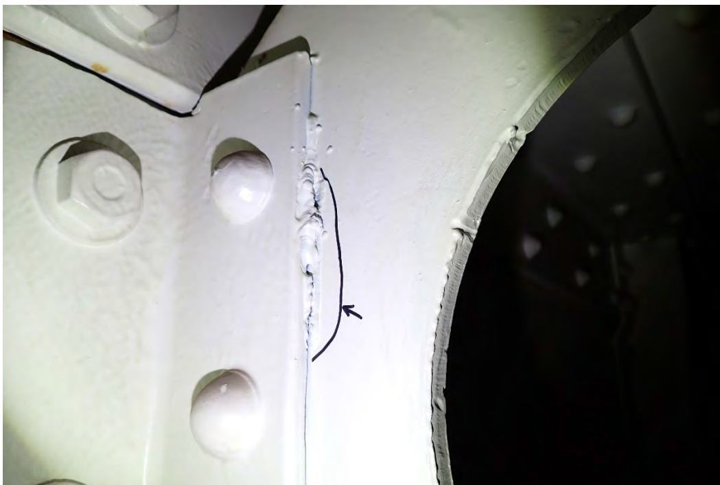
Photo 68 - Typical cracked weld between interior connection bottom angle and the diaphragm plate at Pier 7A, looking northeast.
