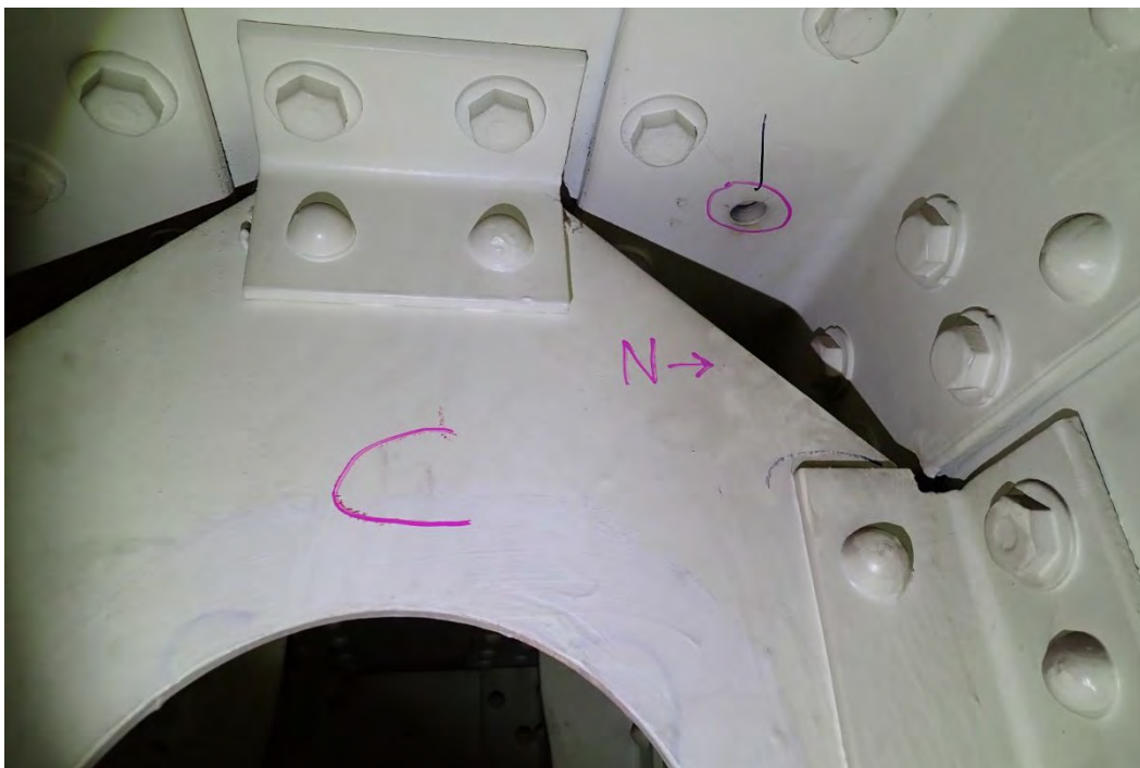
Photo 85 - Top flange angle at Girder C in box cap has a blank hole at Pier 13A, looking west.
