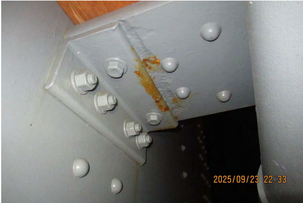
Photo 32 - 1/8" pitting on bottom flange of girder at Pier 6A, looking south. Note: Corrosion has been painted over.
