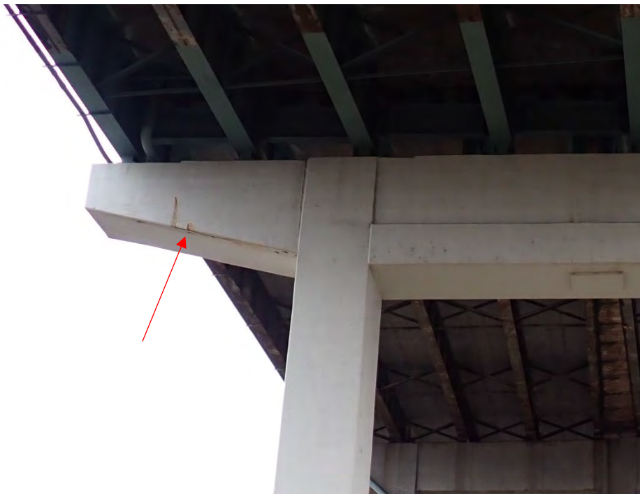
Photo 124 - Transverse cracks with rust staining along the bottom south edge of the west overhang of Pier 19A, looking north
