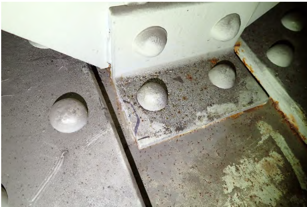
Photo 66 - Typical freckled rust on the surface of the bottom flange plates and bottom flange angles in box cap of Pier 6A.
