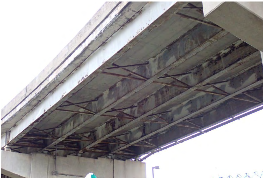
Photo 99 - Span 27B exhibits typical paint failure on girders with chalking, dulling, flaking, and peeling, looking south.
