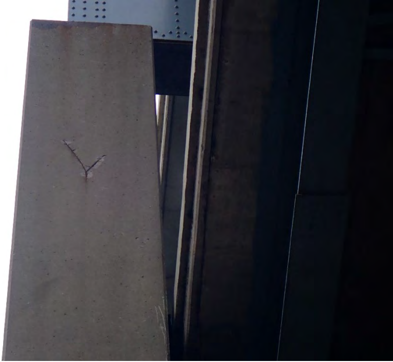
Photo 113 - Minor spalling around rebar on Pier 5A east column, looking south.
