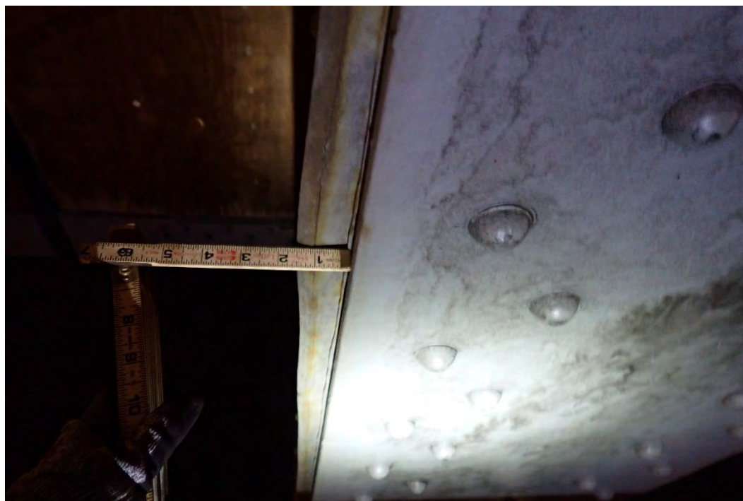
Photo 56 - 1" thick pack rust below the bottom row of rivets, between the web plates and the internal bottom flange connection angles at Pier 4A.
