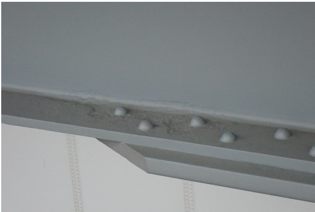
Photo 31 - Typical Painted over minor section loss from previous corrosion on bottom flange at Pier 7A, looking east.
