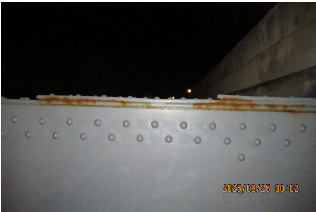
Photo 72 - 3/4" pack rust on top flange cover plates at Girder G of box cap of Pier 9A, looking south.
