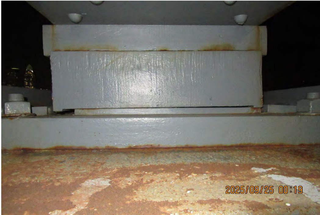
Photo 95 – The upper portion of the bearing has shifted creating a gap between the upper bearing and sole plate of the east bearing of Pier 11A, looking east.
