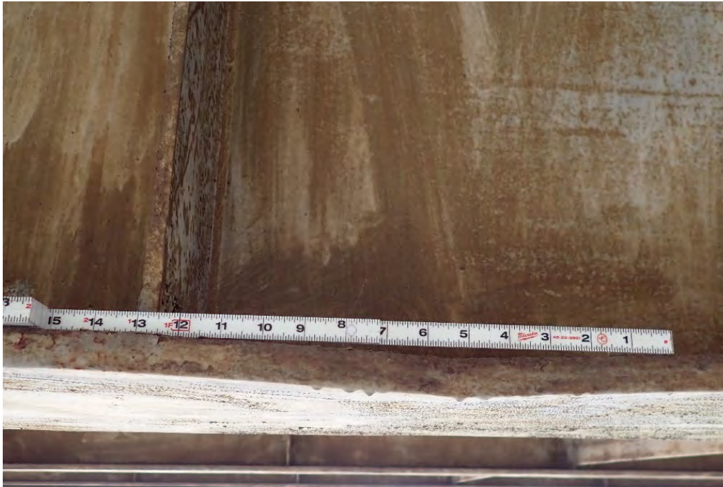
Photo 38 - Bent bottom flange of Girder E of Span 17A, looking west.
