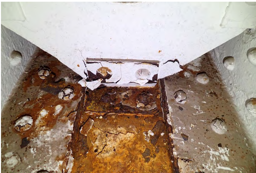
Photo 78 - Section loss with 1/4" of steel thickness remaining on internal diaphragm bottom angle and rivets of Girder G in box cap of Pier 10A, looking east.
