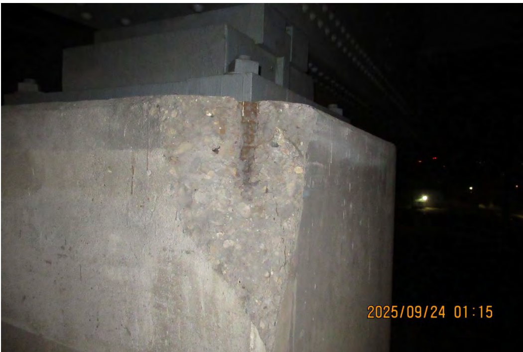
Photo 116 - 12" x 12" x 3" corner spall with exposed rebar at Pier 11A, looking southwest.
