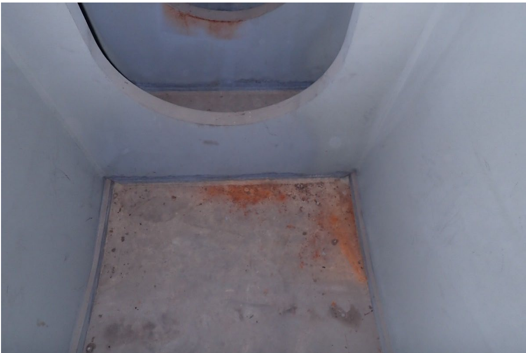
Photo 92 - Minor surface corrosion in box cap interior, at FWW Pier 2, looking north.
