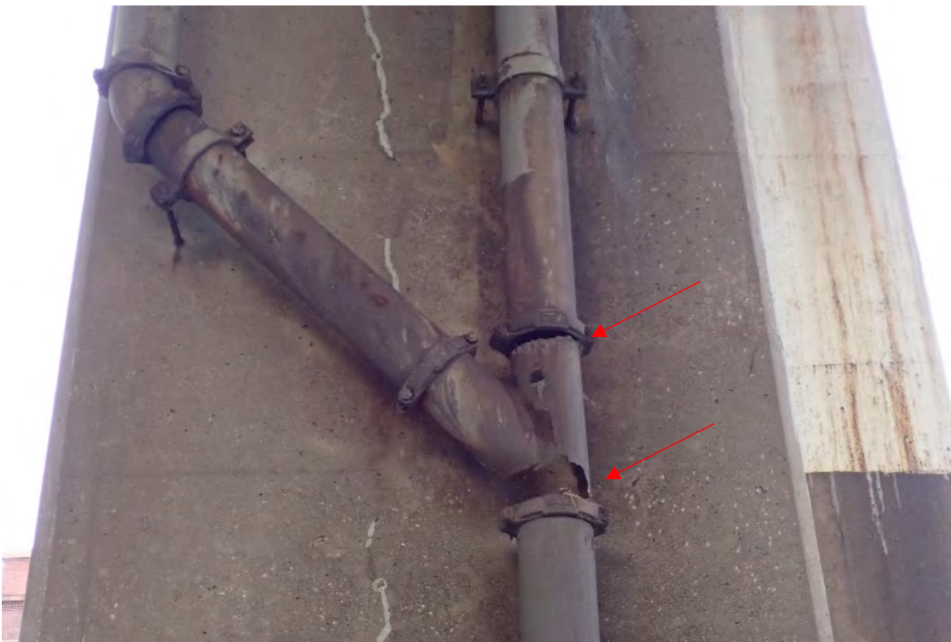
Photo 29 - Corroded drainpipe, with holes and disconnections at joints at River Pier west column, looking west.
