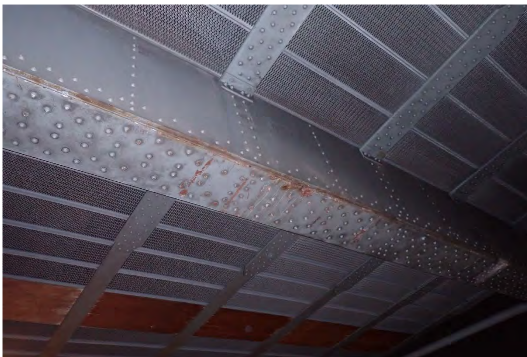
Photo 48 - Typical surface corrosion and impact damage on bottom flange of box cap at Pier 1A, looking northeast.
