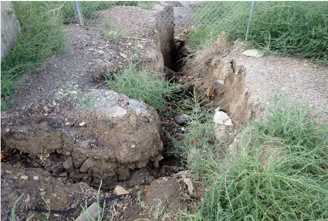
Photo 114 - Up to 24" of erosion at the east column base of Pier 18A, looking south. Note: Erosion starts at the discharge of the pier drain pipe.
