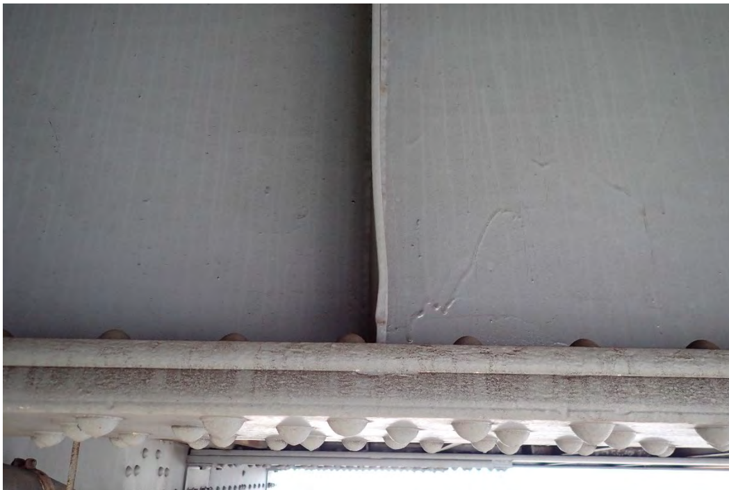
Photo 35 - Typical warped/ bent stiffeners at bottom flange of Girder E Span 13A, looking east.
