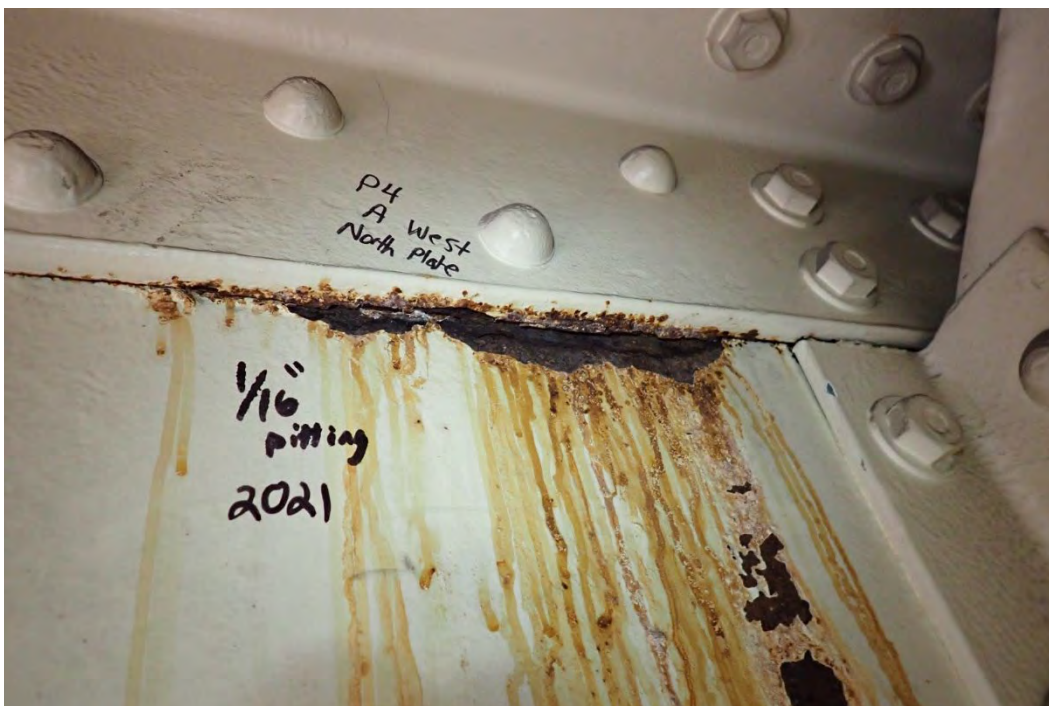
Photo 58 - Typical minor corrosion between the top flange angles, web plates, and filler plates at Pier 4A, looking north.
