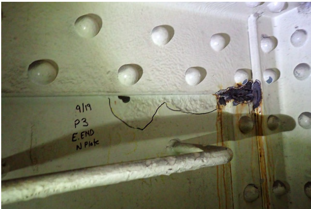
Photo 55 – Painted-over pitting and active corrosion at the east end on Pier 3A, looking north.
