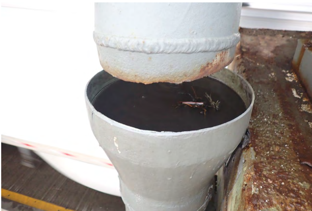
Photo 27 - Typical clogged drainpipe at Pier 8A, looking east.
