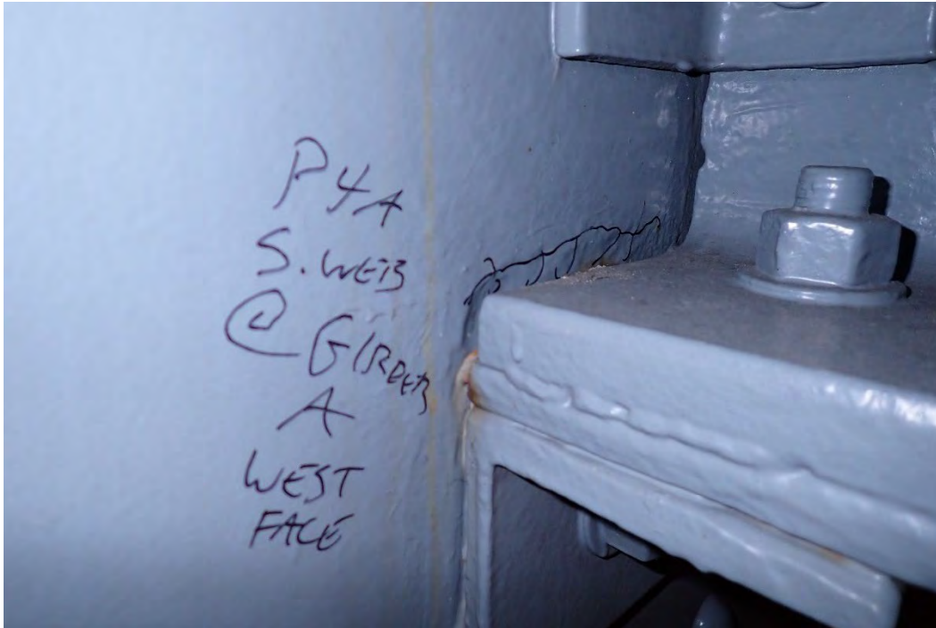
Photo 57 - Up to 1/8" section loss of box cap south web at Girder A seat at Pier 4A, looking north.
