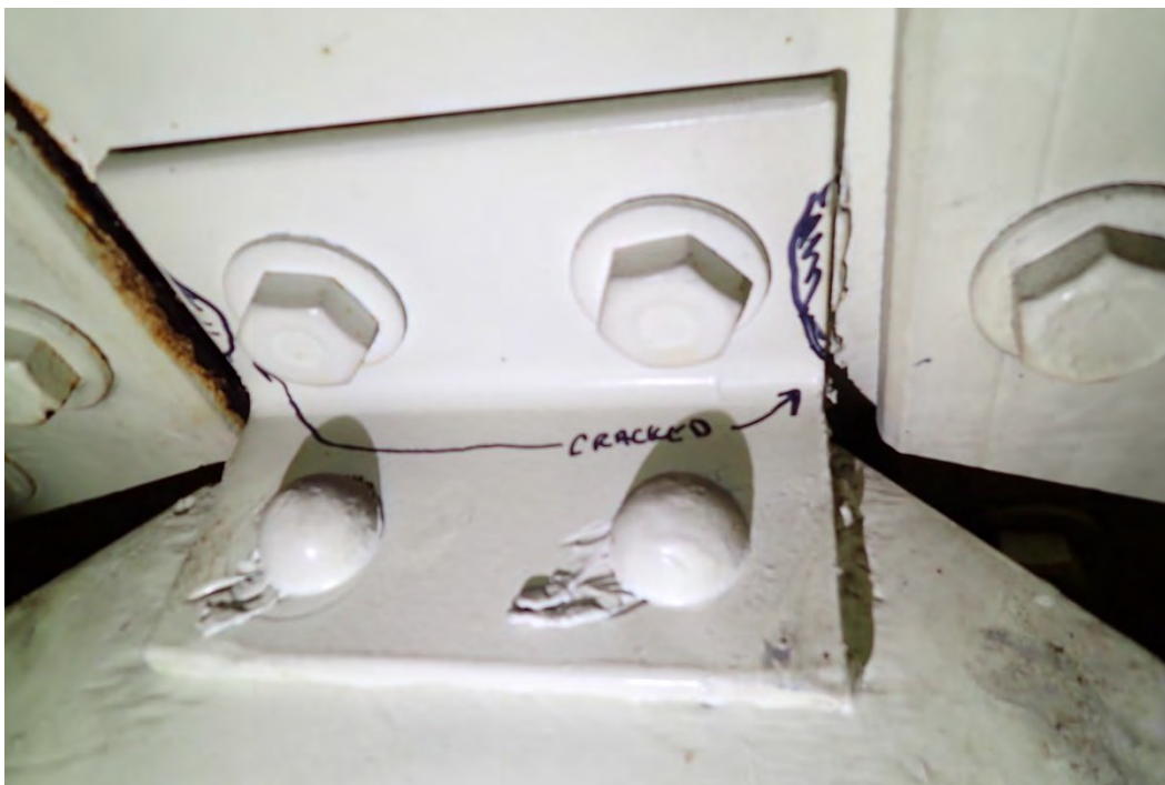
Photo 70 - Cracked welds between the top flange and the top clip angle of the interior diaphragm of Pier 8A, looking west.
