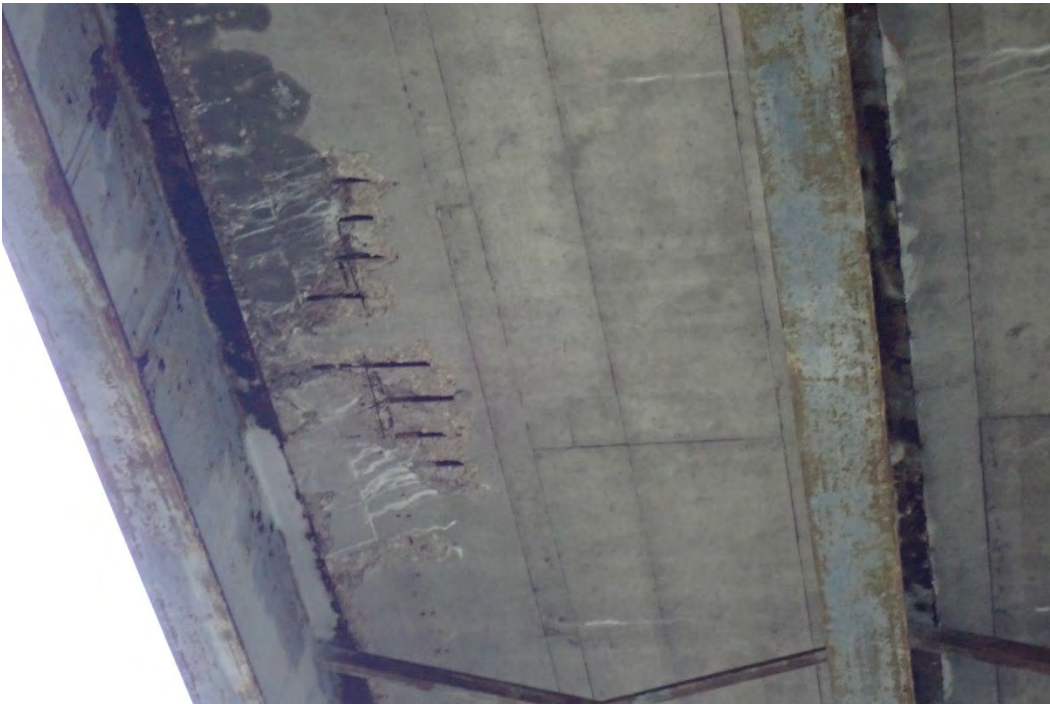
Photo 8 - Typical spalling with exposed rebar on the underside of deck at Span 26B, looking south.
