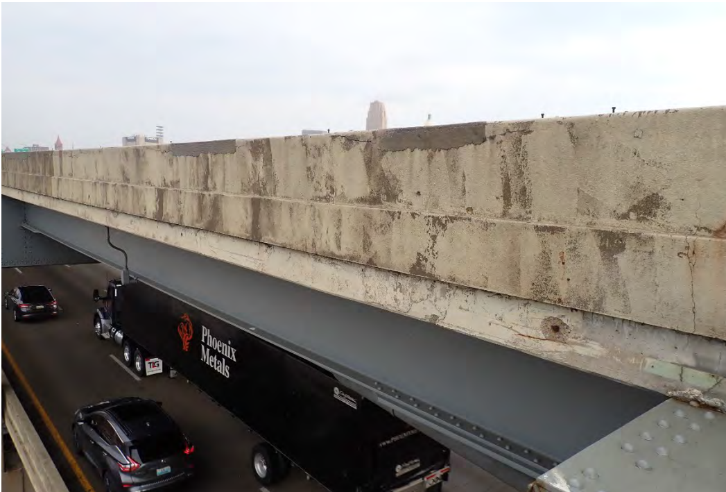
Photo 20 - Typical concrete patch on railing top at Span 3A, looking northeast.
