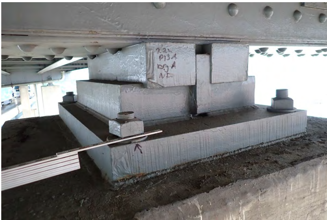
Photo 96 - Bearing nut is backed off at Pier 13A, looking southwest.
