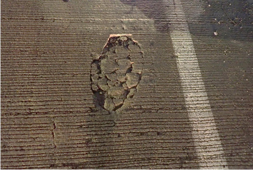
Photo 18 - Pot hole in deck at Span 11A near Pier 10A.
