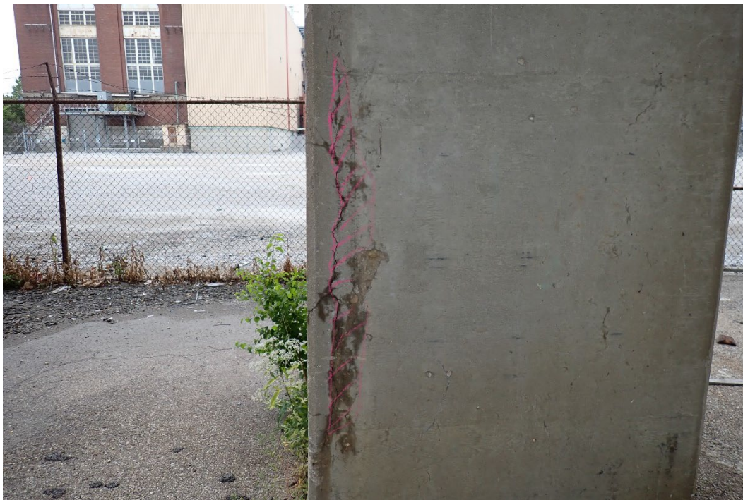
Photo 57 - Minor spalling and delamination on west column of Pier 1A, looking west.
