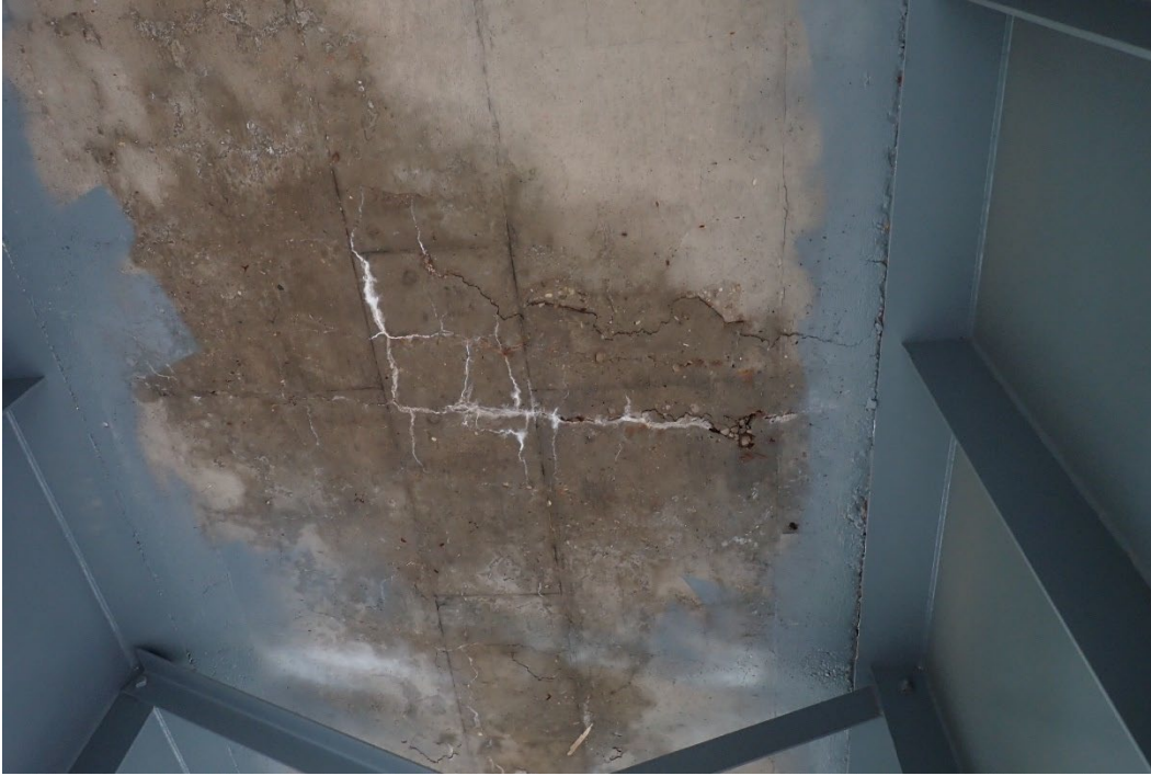
Photo 6 - Delaminated and cracked area with efflorescence, at Span 12A, looking north.
