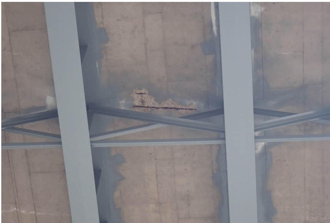
Photo 3 – 2' long x 1' wide deep spall with exposed rebar in Bay 6 of Span 10A, looking south.
