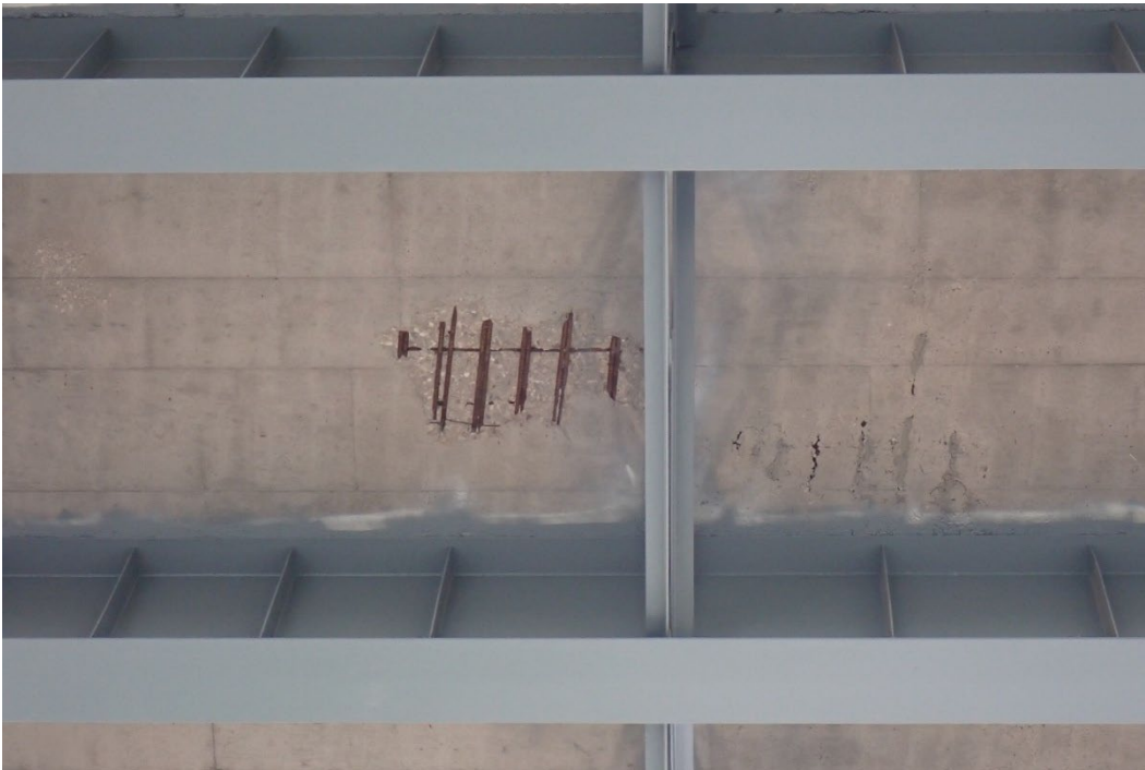
Photo 5 - Deck spall with exposed rebar at Span 11A in Bay 4.
