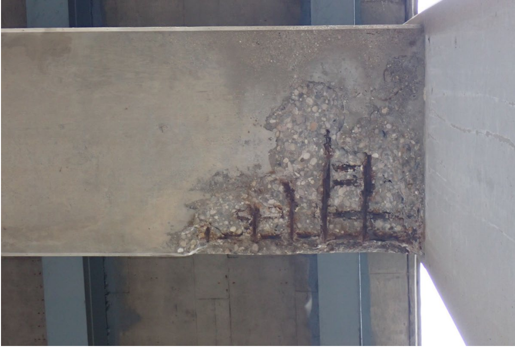
Photo 70 - Large spall with exposed rebar, and delaminated concrete on underside of pier cap at Pier 5A, looking north.
