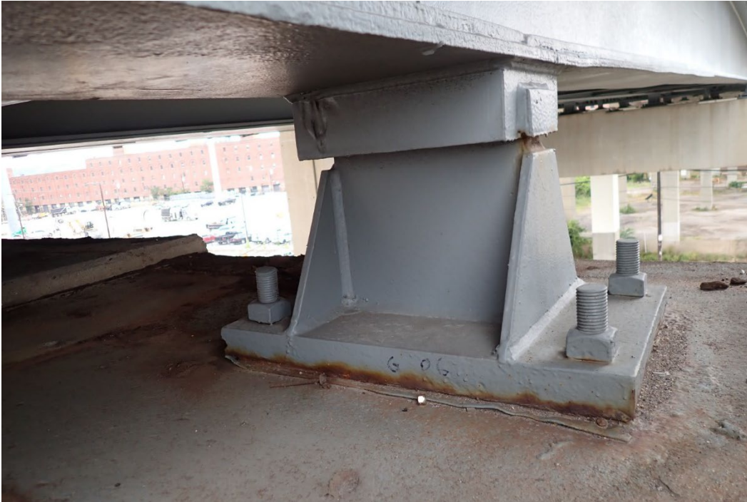
Photo 46 - Typical fixed bearing with minor freckled rust at base, Girder G of Pier 6A, looking north.
