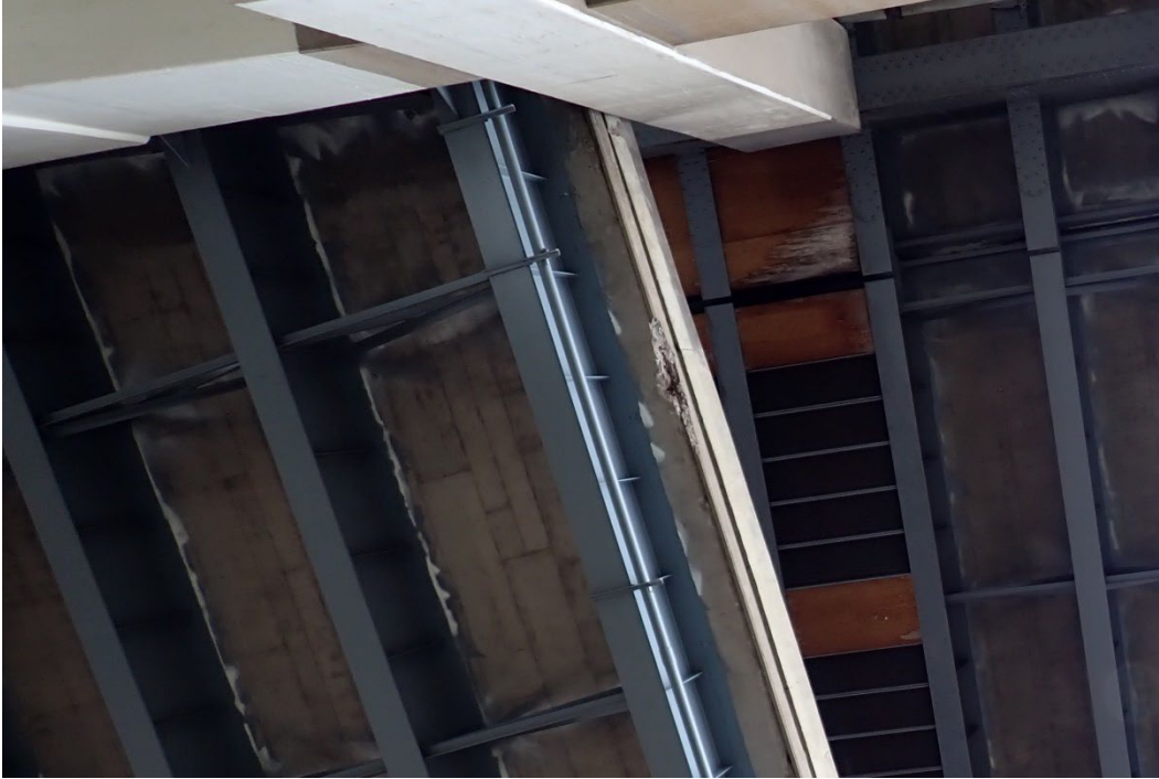
Photo 10 – 4' long spall with exposed rebar on west overhang in Span 12C.
