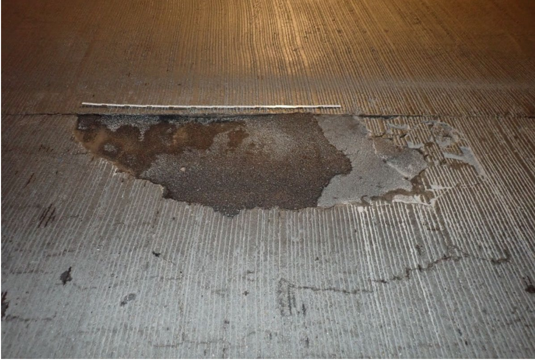
Photo 16 - 10'x 4' asphalt filled pothole in Span 9A near Pier 8A.
