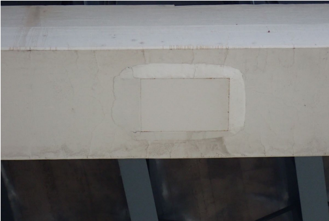
Photo 67 – Steel plate embedded in patched concrete surface of the bottom flange pier cap underside at Pier 12C.
