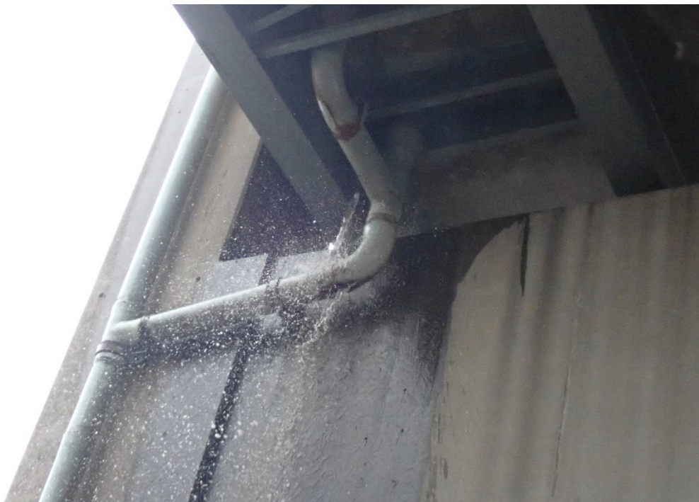
Photo 32 - Clogged and overflowing drainpipe at Pier 2A, looking south.
