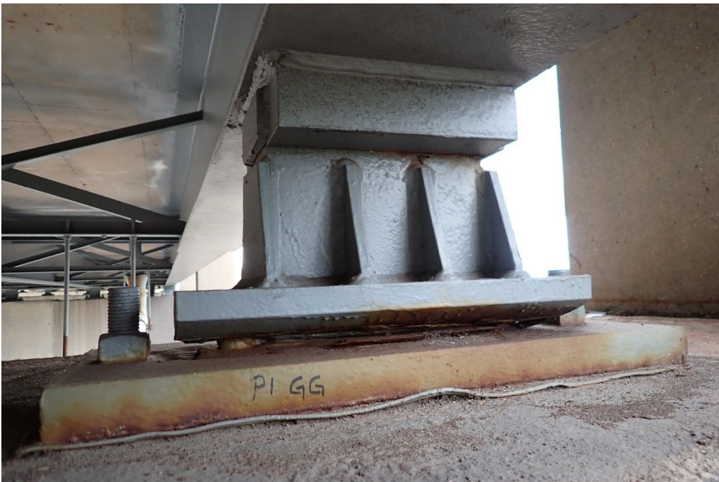
Photo 43 - Rocker bearing with minor surface corrosion at Girder G at Pier 1A, looking north. Note: gap between rocker and sole plate.
