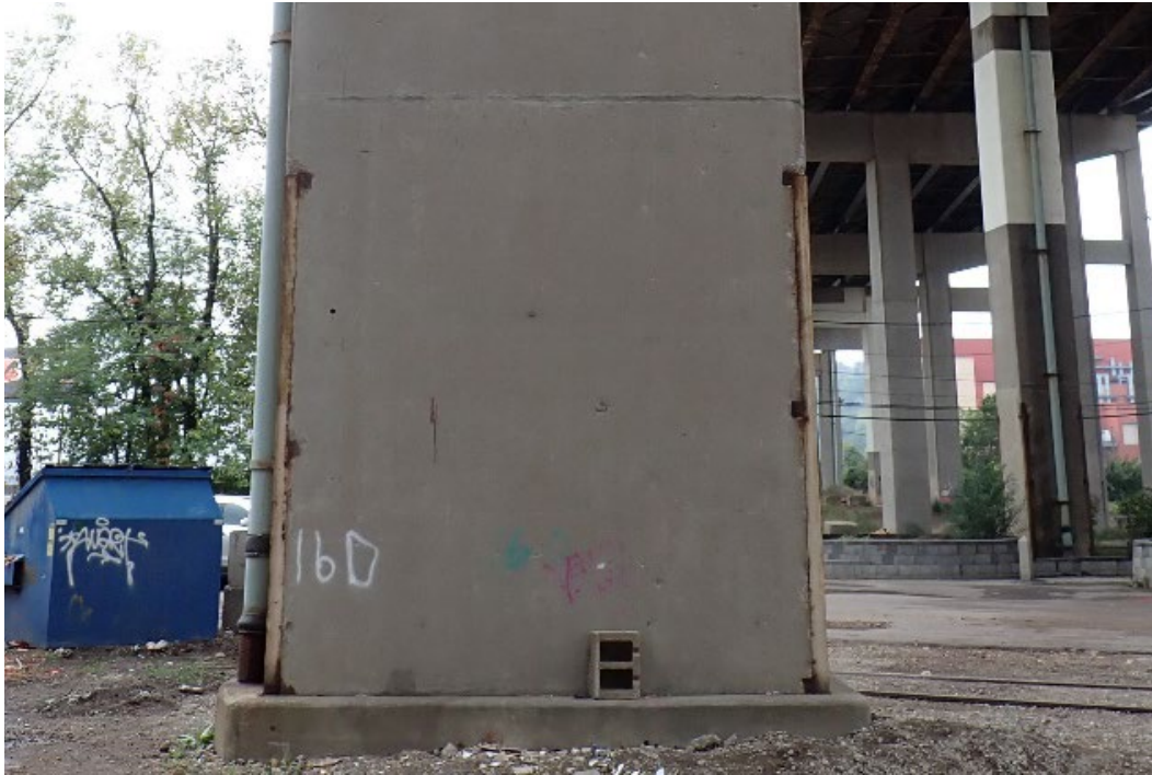
Photo 63 - Minor spalling at corner protection of pier wall at 16D, looking south.
