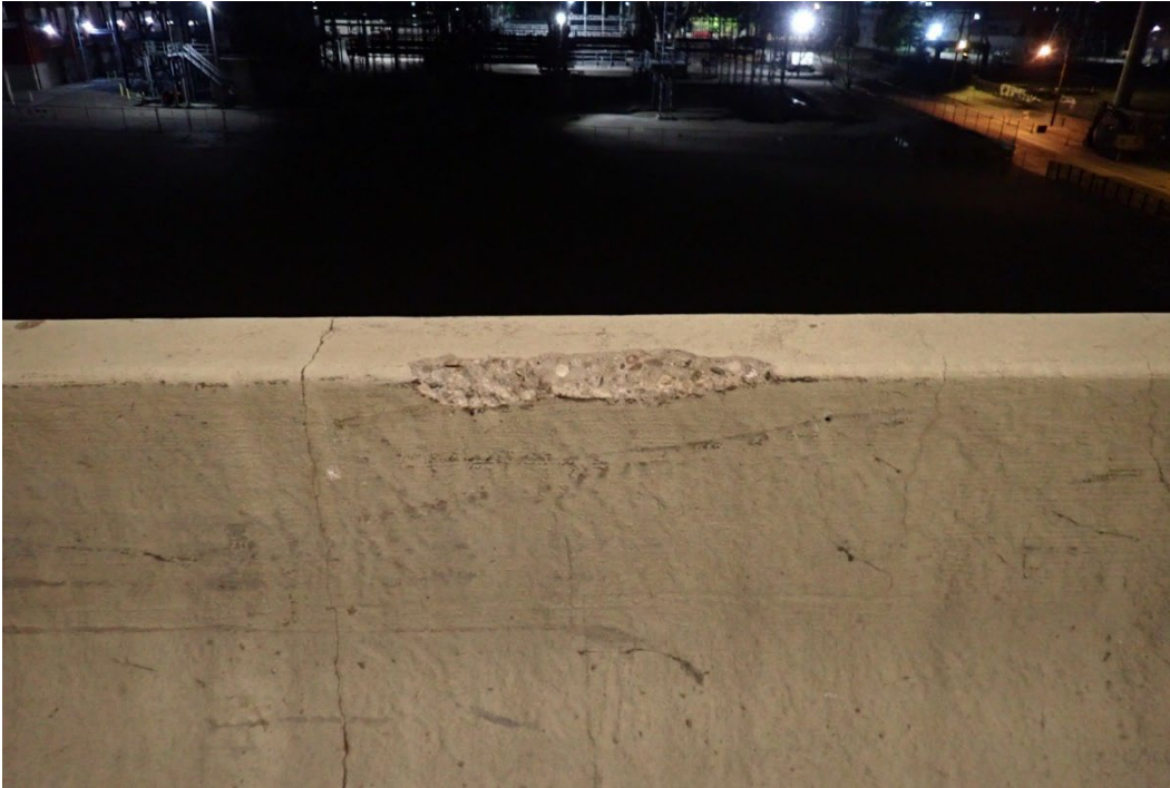
Photo 26 - Minor edge spall on top of west railing a Span 6 mid span looking west.
