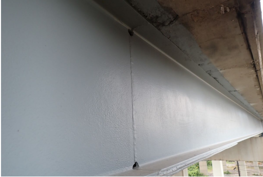
Photo 49 - Typical paint condition for Spans 1A to 13A at fascia Girder G of Pier 6A, looking north.
