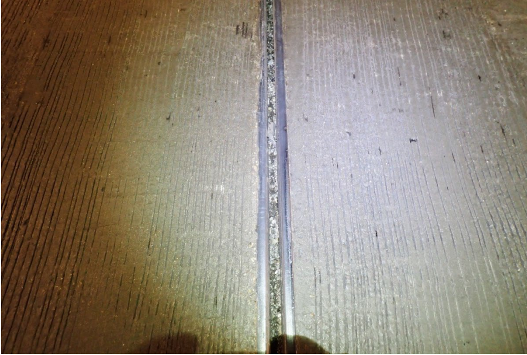
Photo 20 - Typical debris impactation at strip seal joint at Pier 4, looking east.
