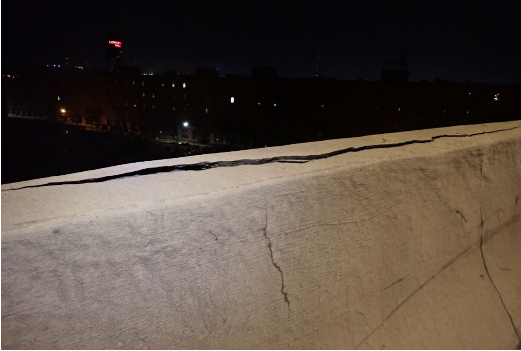
Photo 24 – 6' long corner spalling with delamination on top edge of concrete railing at Span 11A, looking east.
