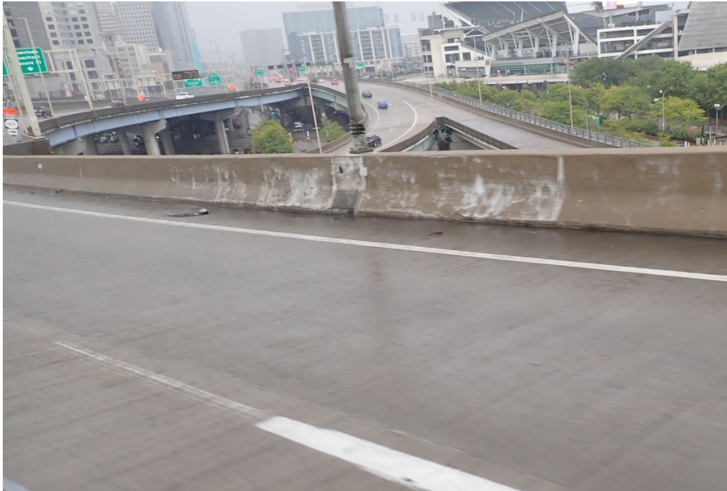
Photo 22 - Hairline longitudinal cracks with efflorescence in concrete railing, looking east.
