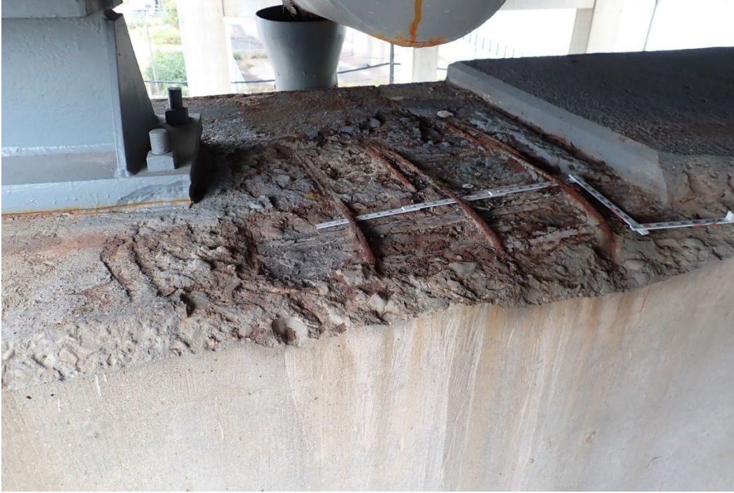
Photo 72 – Large spall with exposed rebar on pier cap Pier 10A, looking south.
