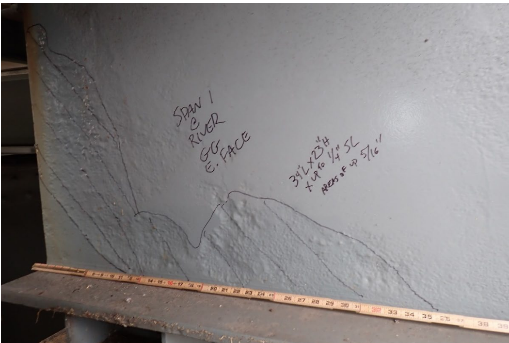
Photo 35 - 34" x 23" x up to 5/16" section loss in web and bottom flange of Girder G at River Pier, looking east.
