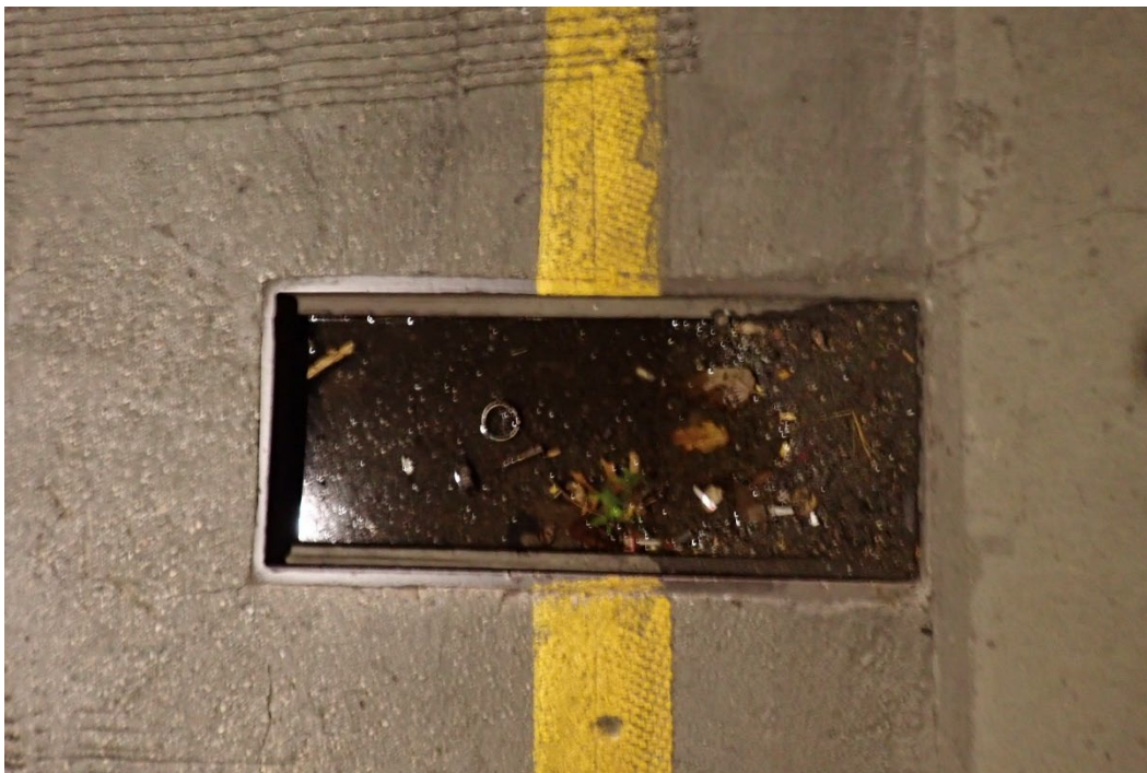
Photo 30 - Missing deck drain grate with debris accumulation, at Span 2A midspan, looking south.
