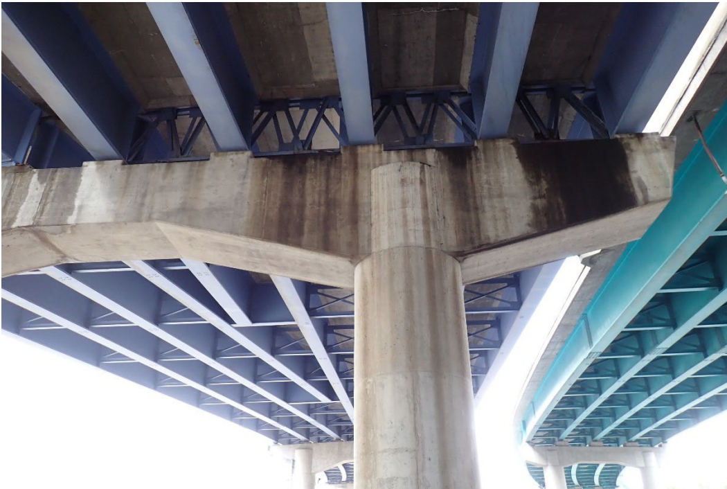
Photo 71 - Joint leaking onto pier cap with staining at Pier 5, looking west.
