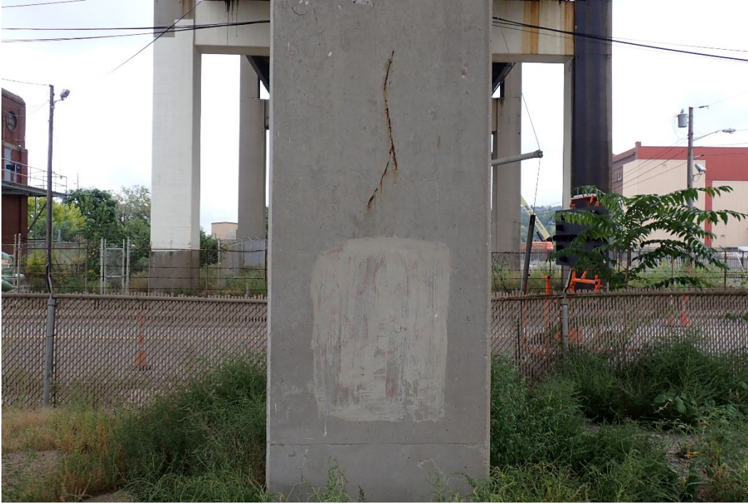
Photo 58 - Minor spall with exposed rebar on middle column of Pier 9A, looking south.
