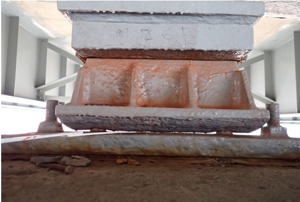
Photo 44 - Rocker bearing with gap up to 1/4" wide with rust fretting at Pier 8A Girder D, looking north.
