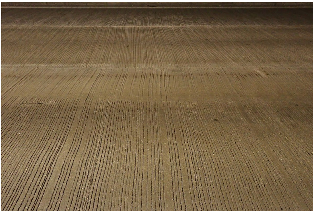
Photo 11 - Typical wearing surface with small spalls and gouges, in Span 6A.
