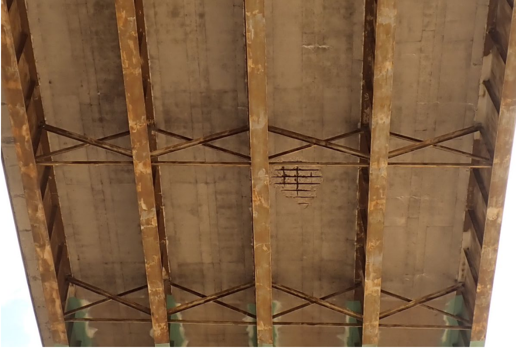
Photo 8 – 64" x 52" x 2 1/2" with exposed rebars in Bay 3 of Span 20D, looking east.
