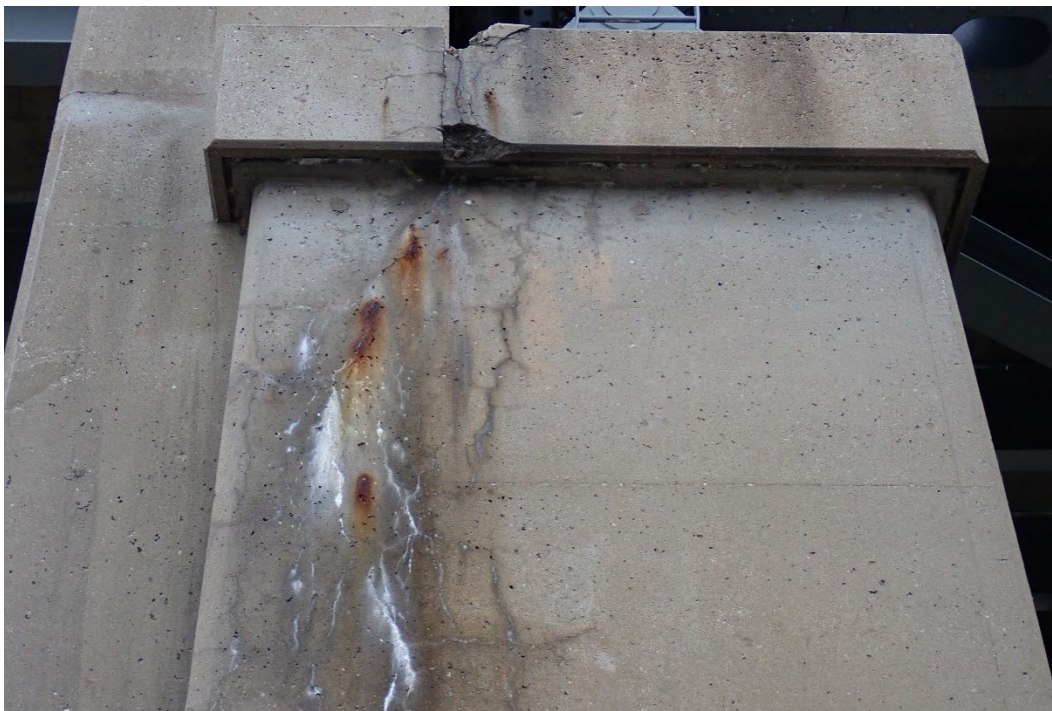
Photo 61 - Map cracking with delamination, efflorescence, and rust staining on west side of River Pier, looking east.
