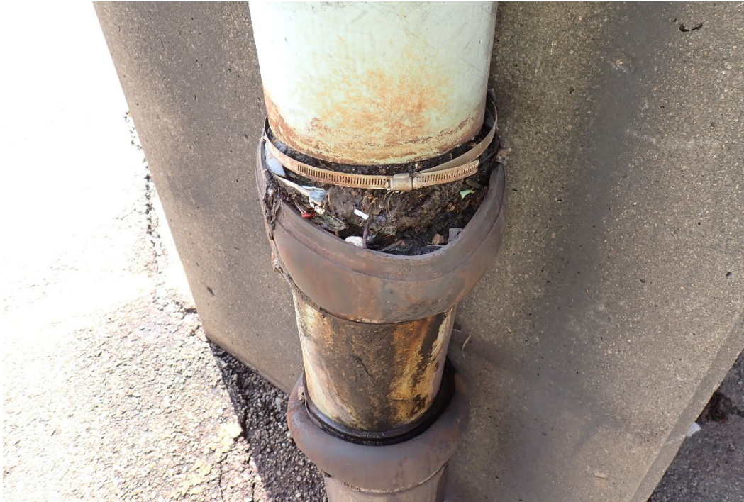
Photo 29 - Drain pipe fully impacted with debris and disconnected at base at Pier 19D, looking west.
