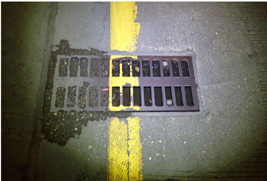
Photo 28 – Typical clogged deck drain at Pier 1, looking north.
