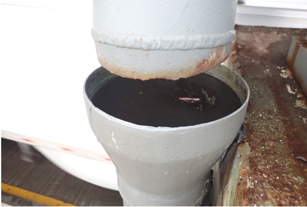
Photo 31 - Typical clogged drainpipe at Pier 8A, looking east.
