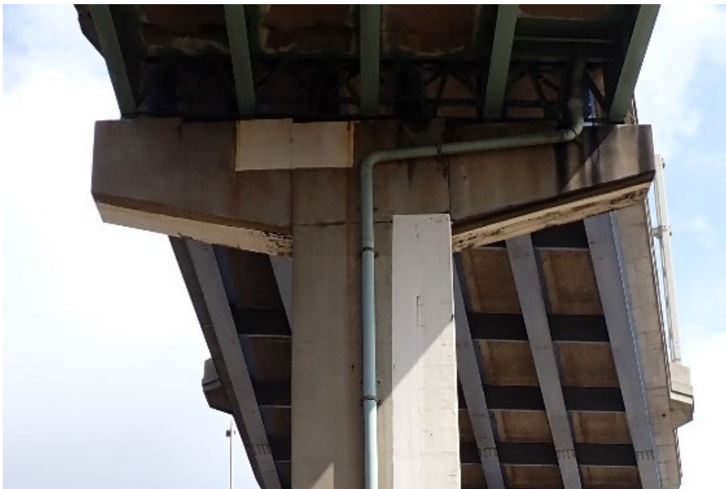
Photo 69 - Minor cracking on the pier cap overhangs on Pier 20D, looking east.
