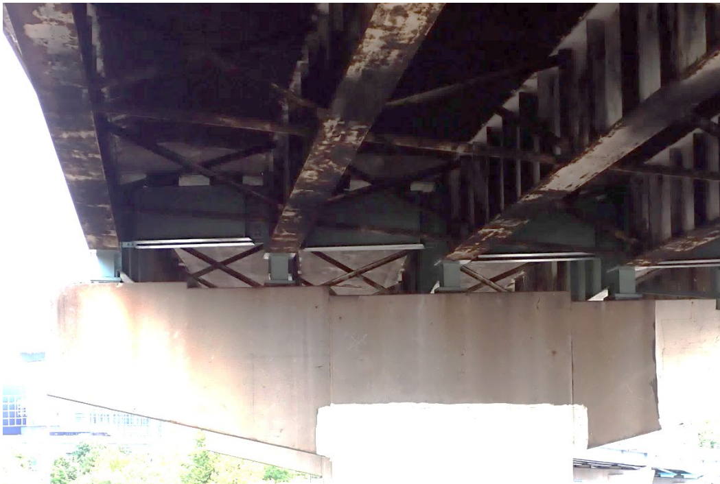
Photo 48 - Typical coating condition for Spans 15C to 20D, at Span 17D, looking east. Note: failed coating system with chalking, dulling, flaking, peeling, and surface corrosion.
