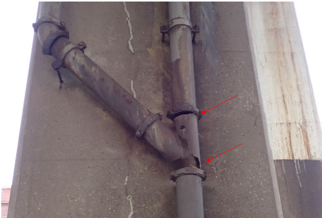
Photo 33 - Corroded drainpipe, with holes and disconnections at joints at River Pier west column, looking west.
