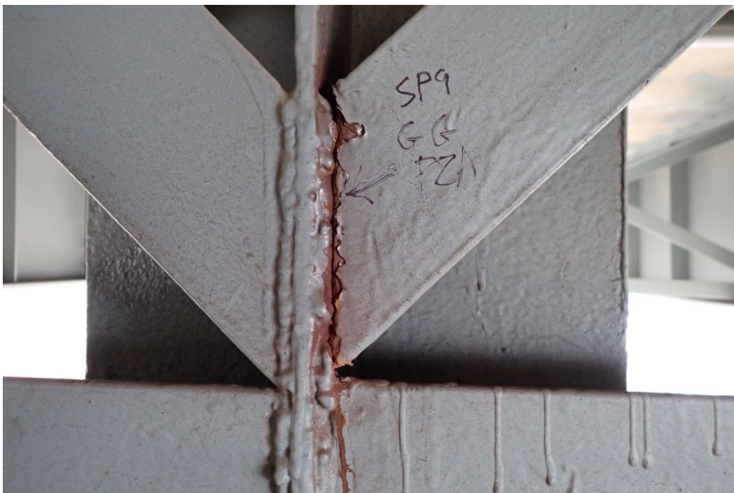
Photo 54 - Broken weld at end of cross frame of Girder G in Span 9A, looking north.
