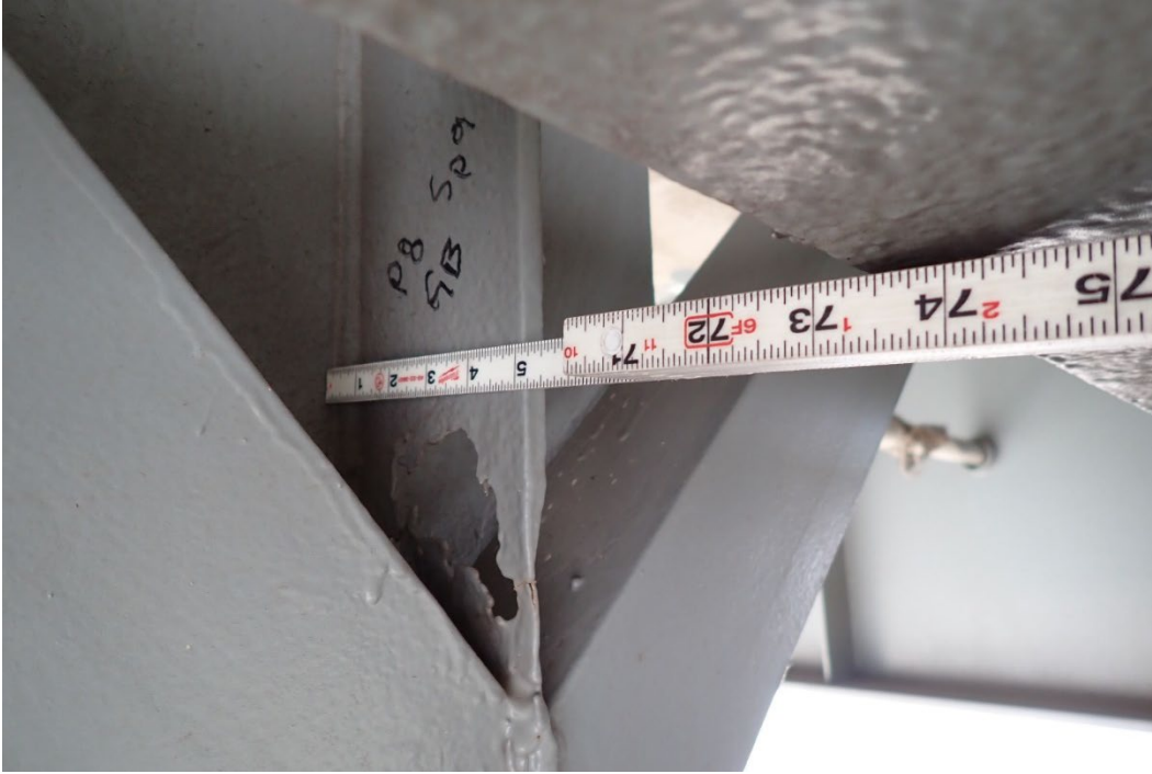
Photo 38 - Corrosion hole in beam web at Pier 8A Girder B, looking northeast.
