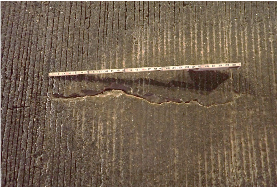
Photo 17 - Moderate crack to deck in Span 10A near Pier 10A.
