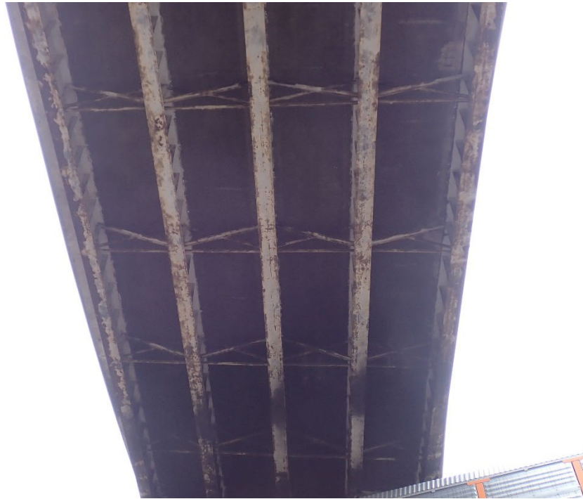
Photo 1 - Soot staining the underside of Span 17D, looking north.
