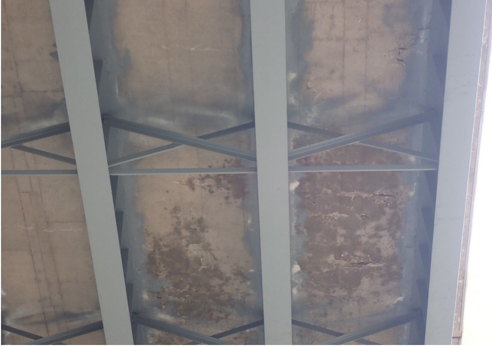
Photo 4 - Minor spalls with exposed rebar in Bay 7 of Span 10A, looking south.
