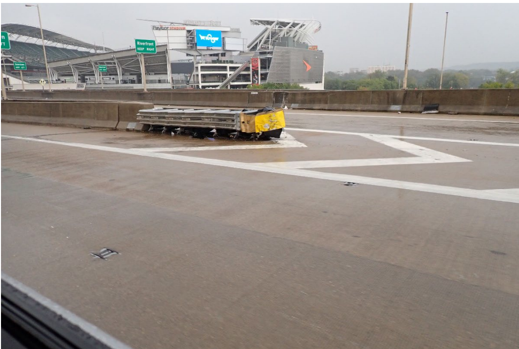
Photo 27 - Minor damage to impact attenuator at I-71 & 2nd street split, looking south.
