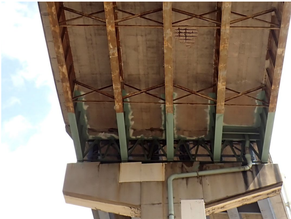
Photo 50 - Typical deck joint location where the superstructure steel was recently painted, at Pier 20D, looking east.
