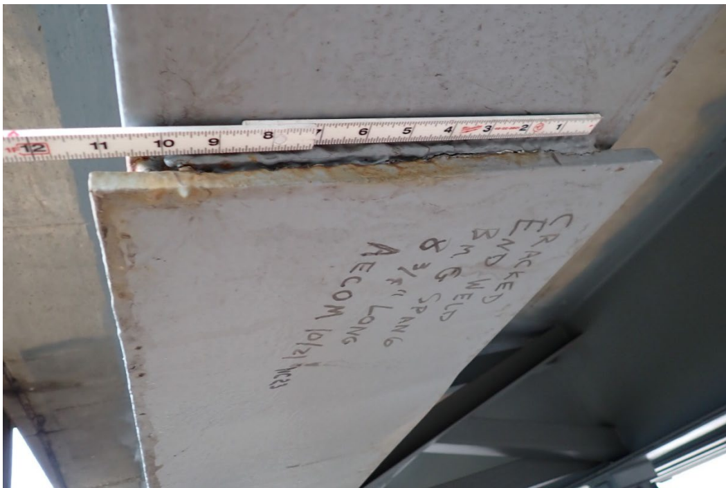
Photo 37 - Cracked cover plate on Girder G in Span 6, looking south.
