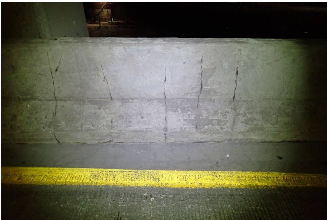
Photo 23 - Typical hairline vertical cracking on bridge railing at west railing at River Pier, looking west.
