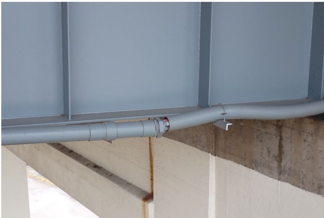
Photo 73 - Separated conduit expansion connection, at Span 7A, near Pier 6A, looking south.
