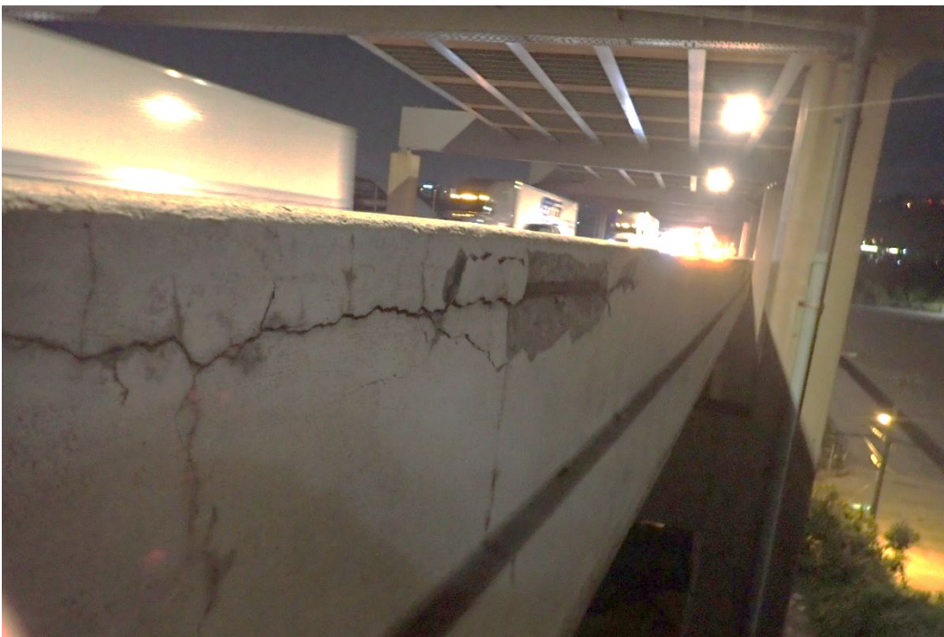
Photo 25 - Longitudinal cracking, with delamination on outside of concrete railing at Span 11A, looking north.
