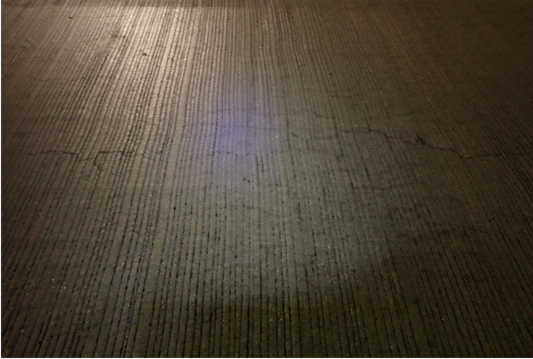
Photo 12 - Typical isolated longitudinal cracking in wearing surface at Span 10A.
