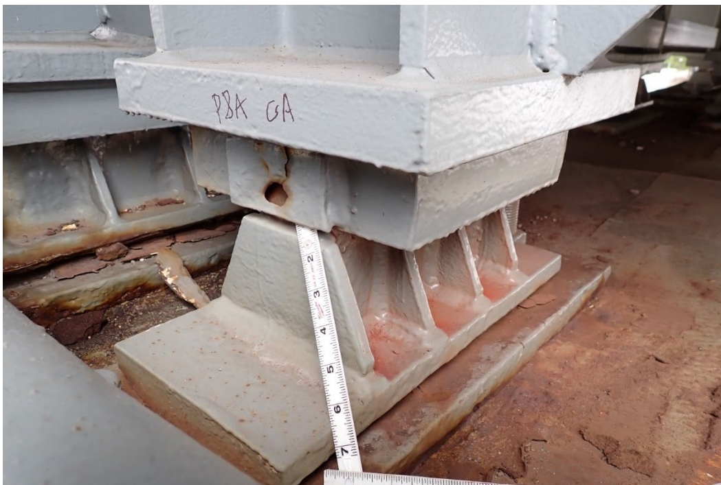
Photo 45 - Hole in bearing keep plate at Girder A of Pier 8A, looking northeast. Corrosion hole in bearing keeper plate at Girder A of Pier 8A, looking northeast.
