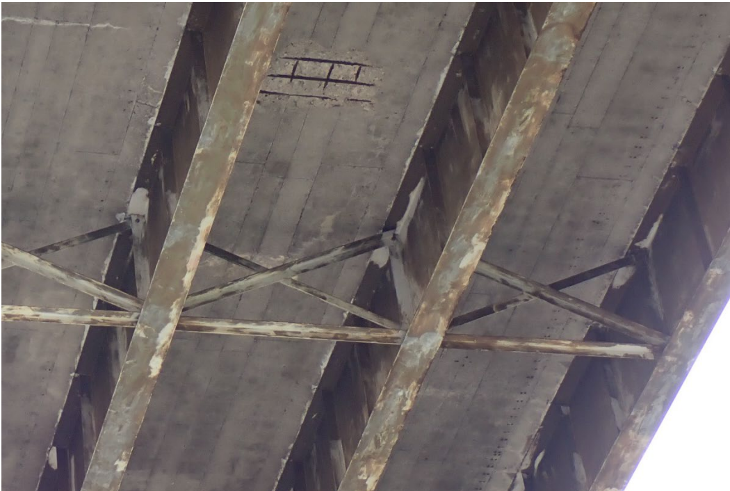
Photo 7 – 36" x 48" x 2 1/2" spall with exposed rebar in Bay 2 of Span 18D.
