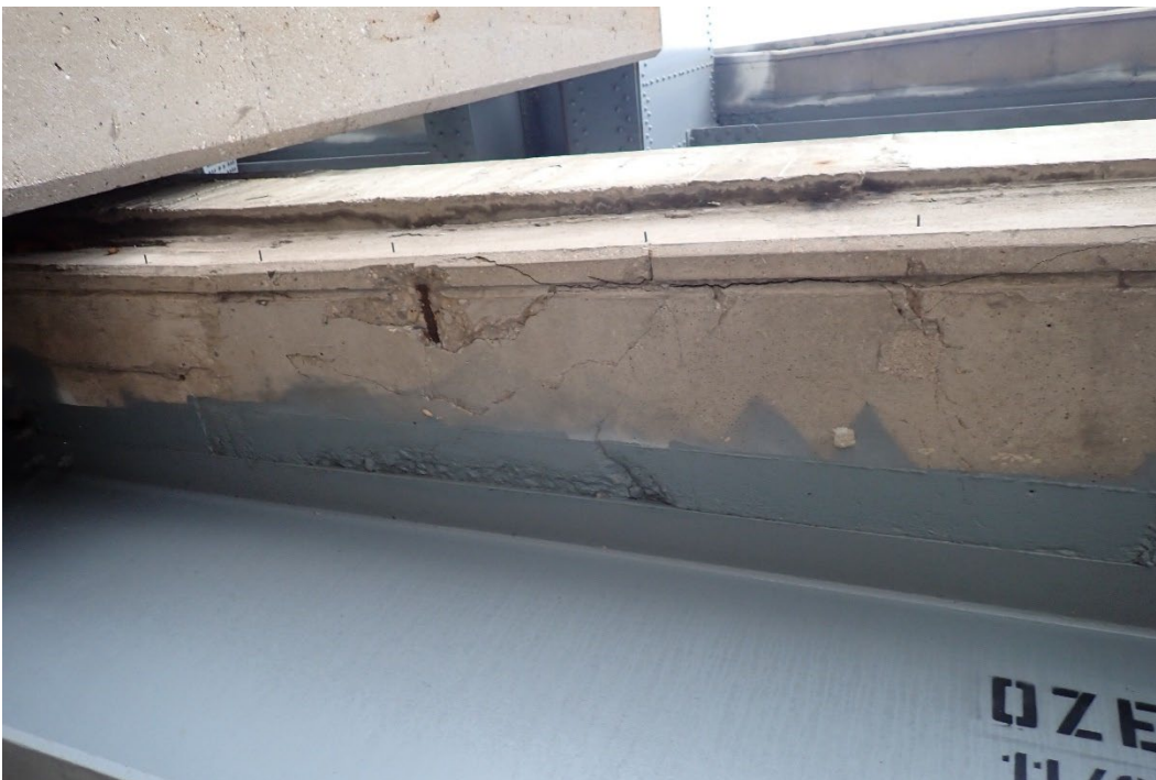
Photo 9 - Spall with exposed rebar under parapet in Span 1A.
