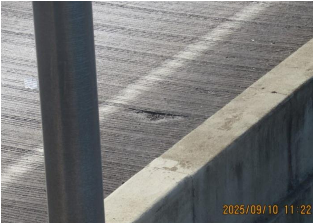
Photo 7: 1'L x 6"W x 1" deep spall in west shoulder (Span 23A)
