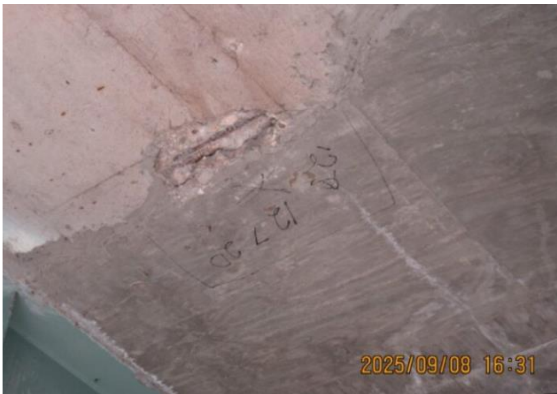
Photo 2: 1'L x 6"W x 2" deep spall with exposed rebar near Pier 19A (Span 20A)
