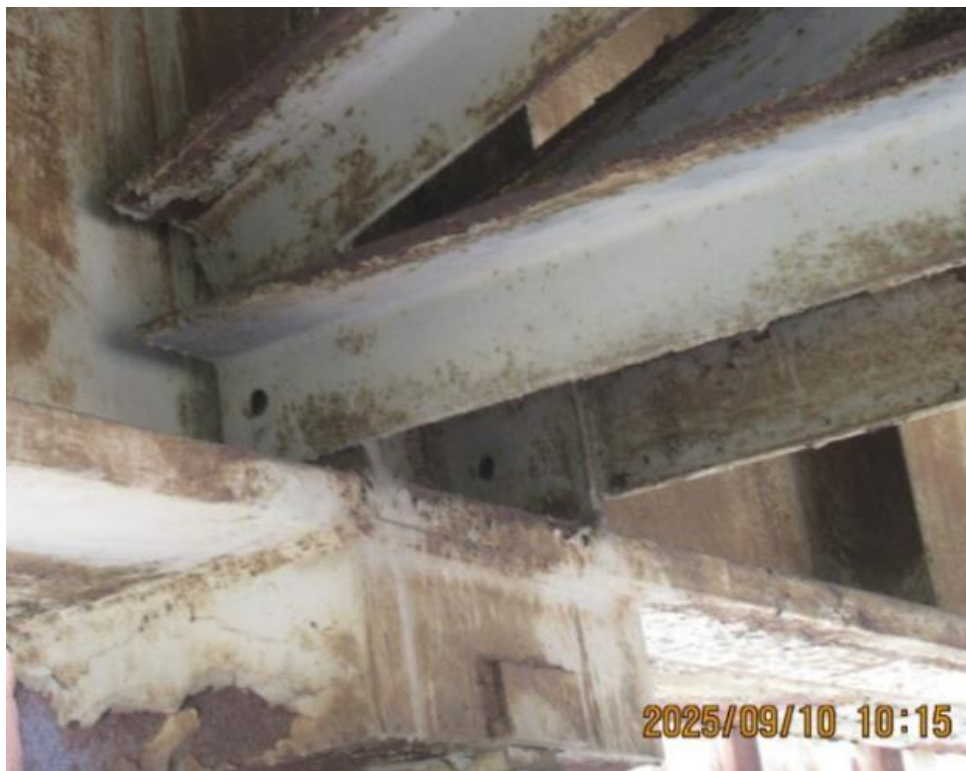
Photo 29: Missing crossframe bolts at Girder E (Pier 21A)
