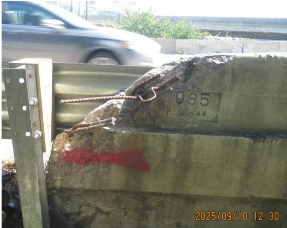
Photo 21: Full width x full height x 3' long spall with exposed and deformed reinforcement
