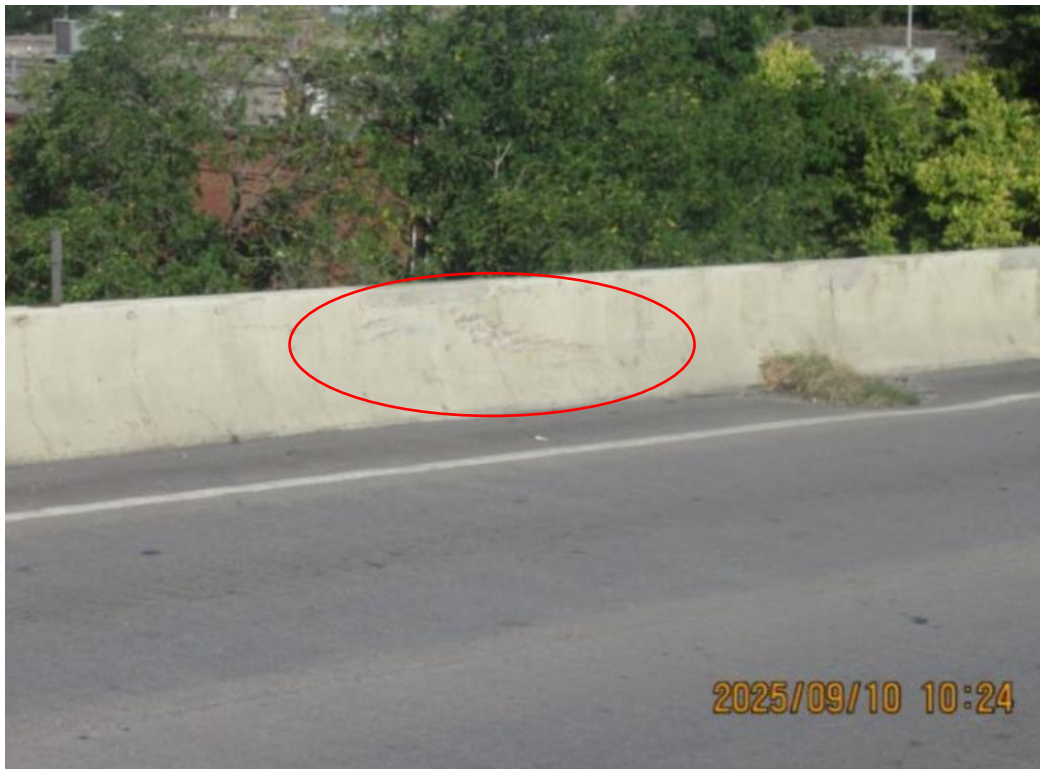
Photo 19: 5'L x 1'H x 1" deep spall due to impact damage railing (Span 22A shown)
