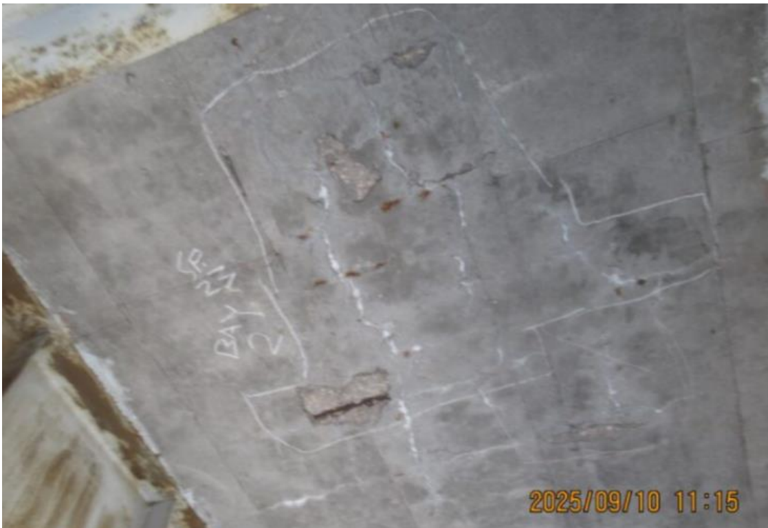
Photo 4: 8'L x 8'W x 1" deep area of spalling and delamination (Span 22A)
