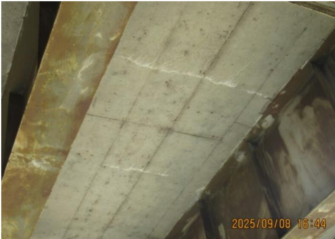
Photo 1: Typical transverse crack with efflorescence (Span 20A shown)
