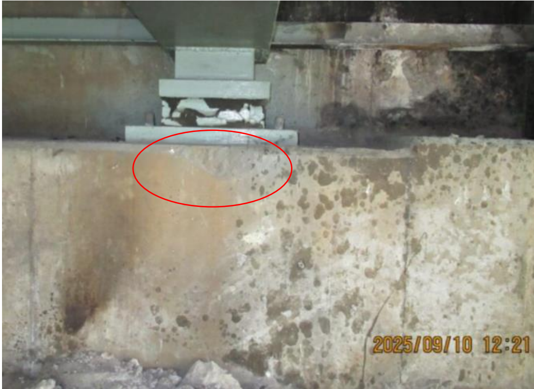
Photo 16: Typical spalling/delamination under bearings (Abutment A)
