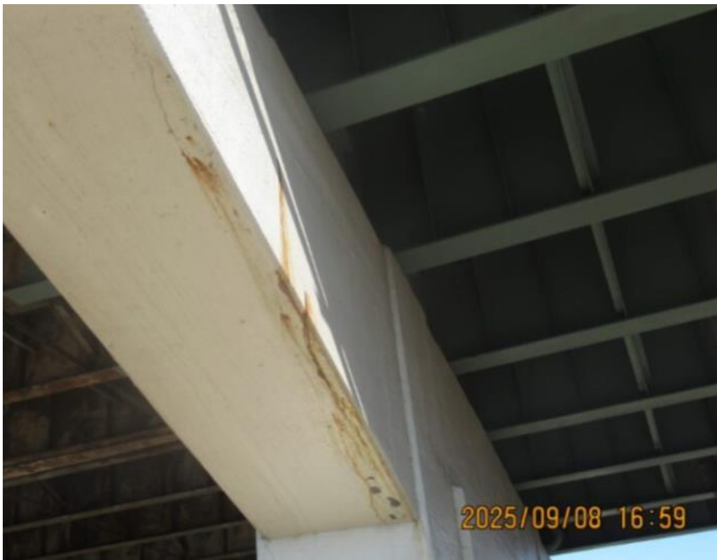
Photo 18: 10'W x 1'L delamination with cracking and rust staining (Pier Cap 19A)
