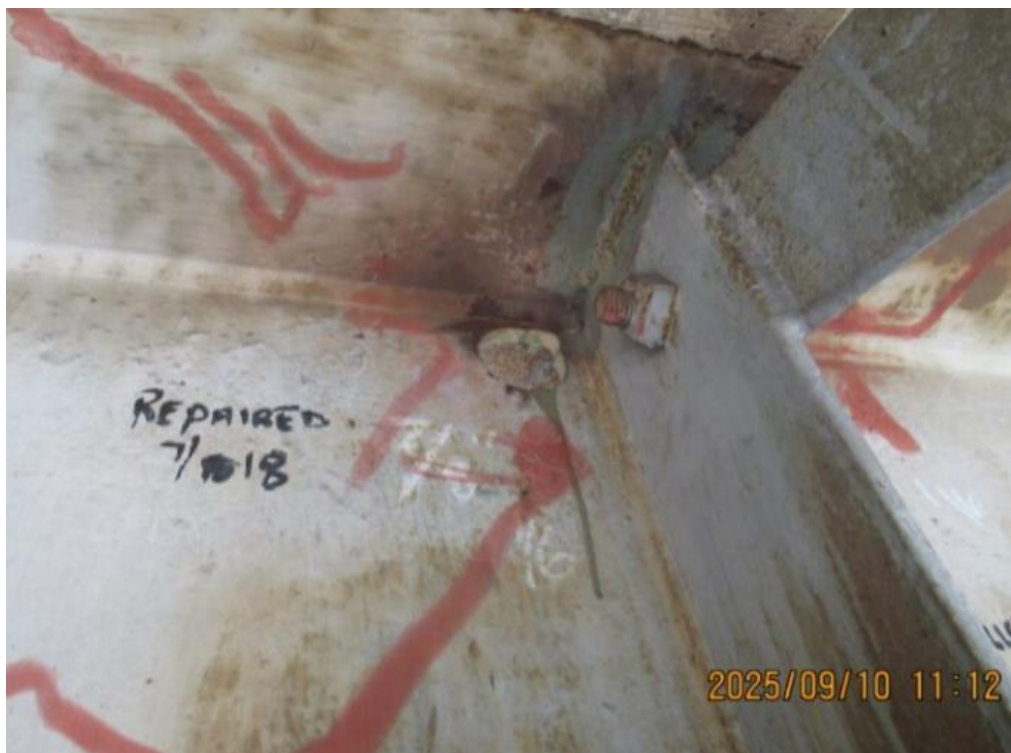
Photo 10: Crack arrest hole in Girder C (Span 23A)
