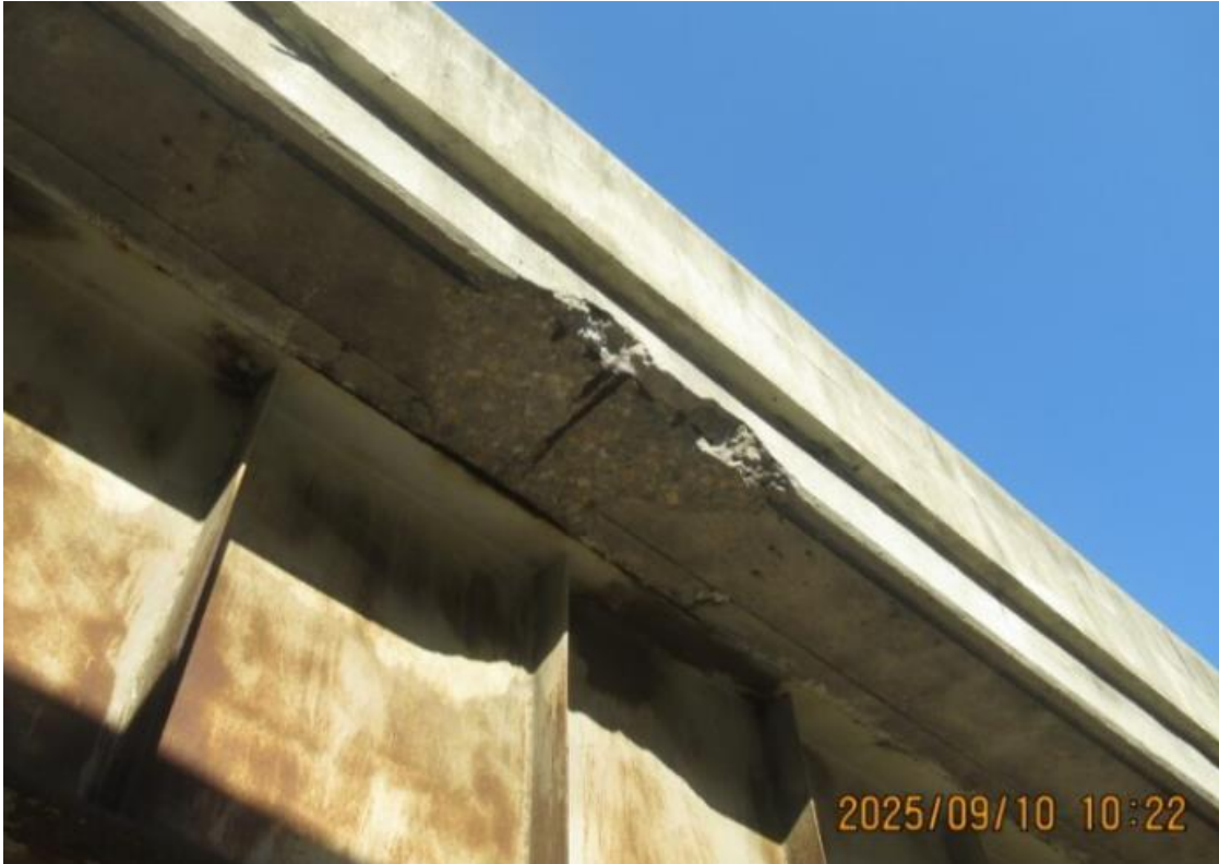
Photo 3: 3'L x 2'W x 4" deep spall with exposed rebar in east overhang (Span 22A)
