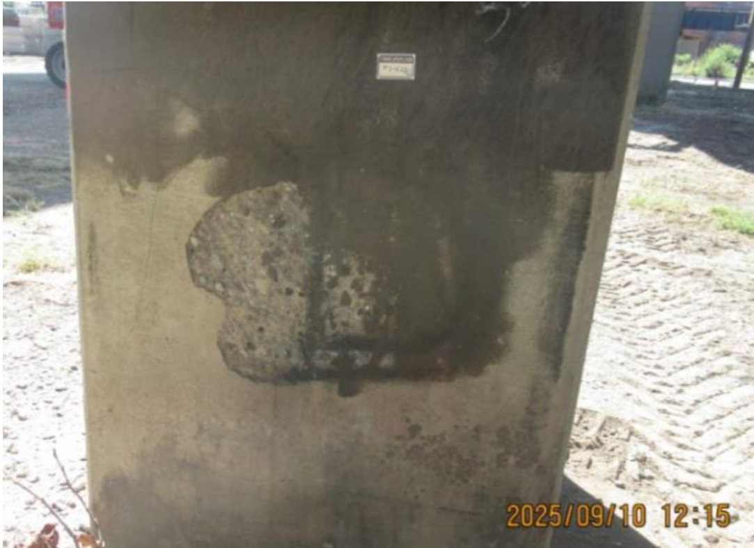
Photo 13: 20" dia. x 1" deep spall on the north face of Column 2 (Pier 23A)
