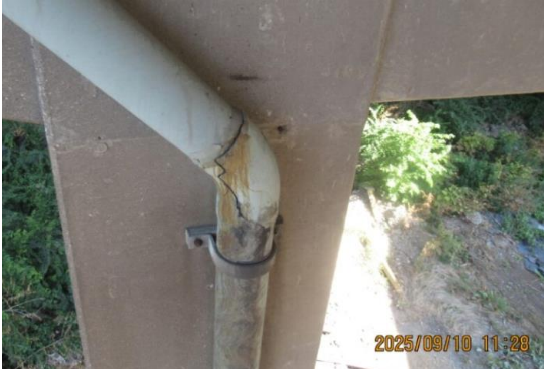
Photo 27: Cracked drainpipe at Column 1 (Pier 23A)
