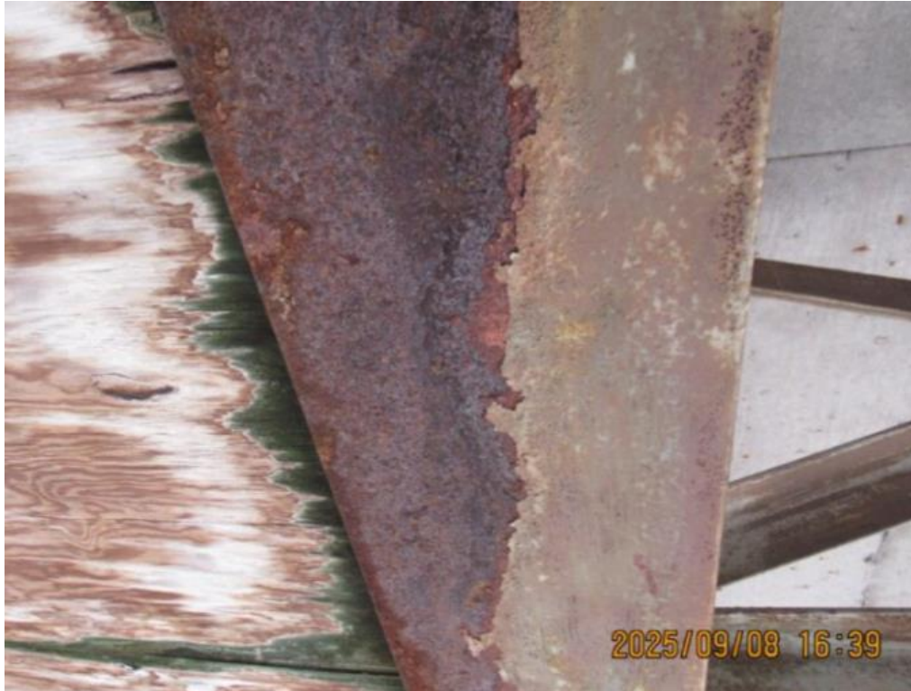
Photo 9: 1/8" deep section loss on west edge of bottom flange of Girder E (Span 20A)
