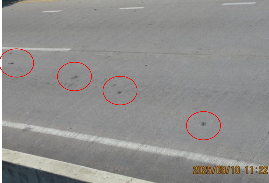
Photo 8: Four shallow spalls up to 4" in dia. in west lane (Span 24A)
