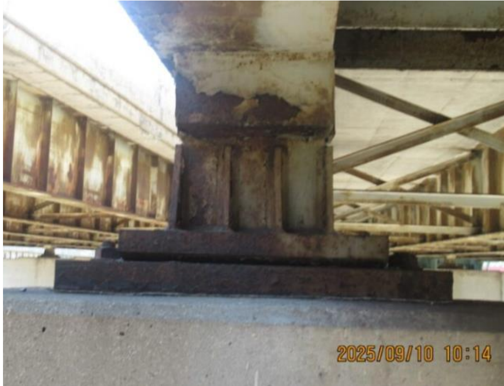
Photo 22: Typical surface corrosion on bearings (Bearing E, Pier 21A)
