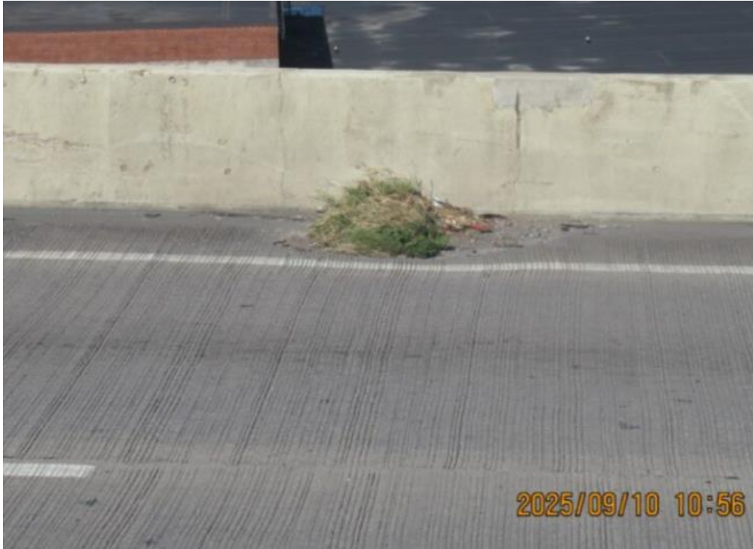
Photo 25: Typical clogged scupper with debris accumulated over top (Span 23A)
