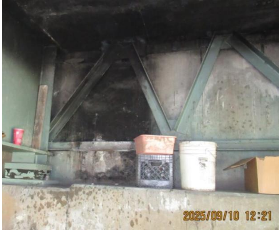
Photo 28: 3' long area of damage along the bottom horizontal member (Abutment A)
