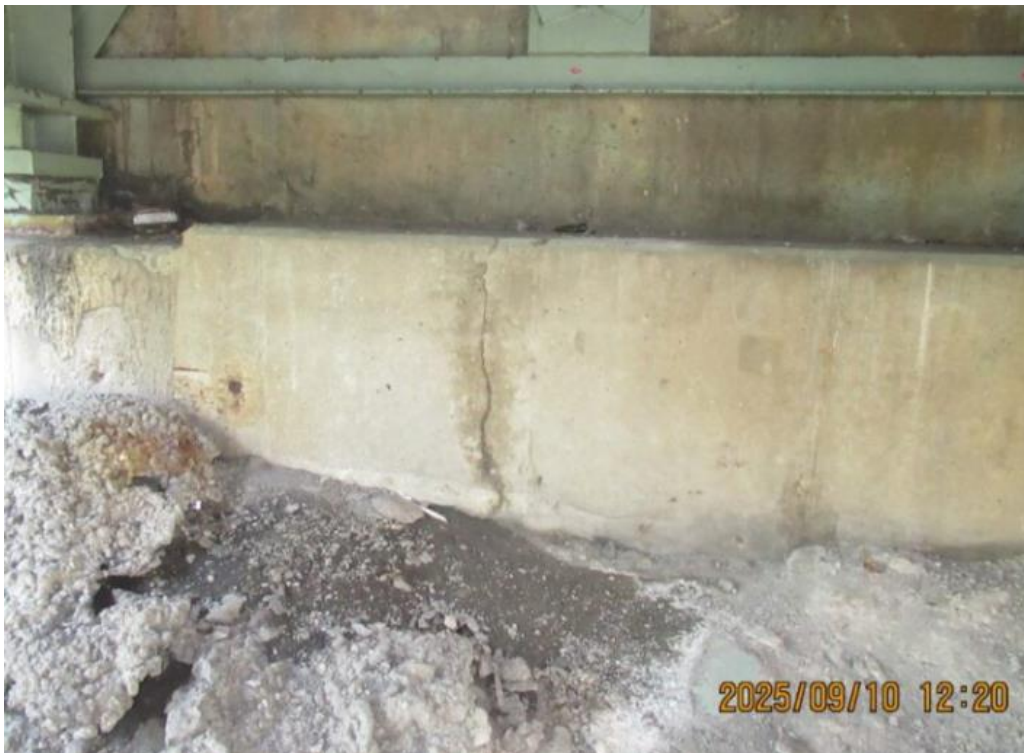
Photo 15: Full height vertical crack between Bearings A and B (Bay 1, Abutment A)
