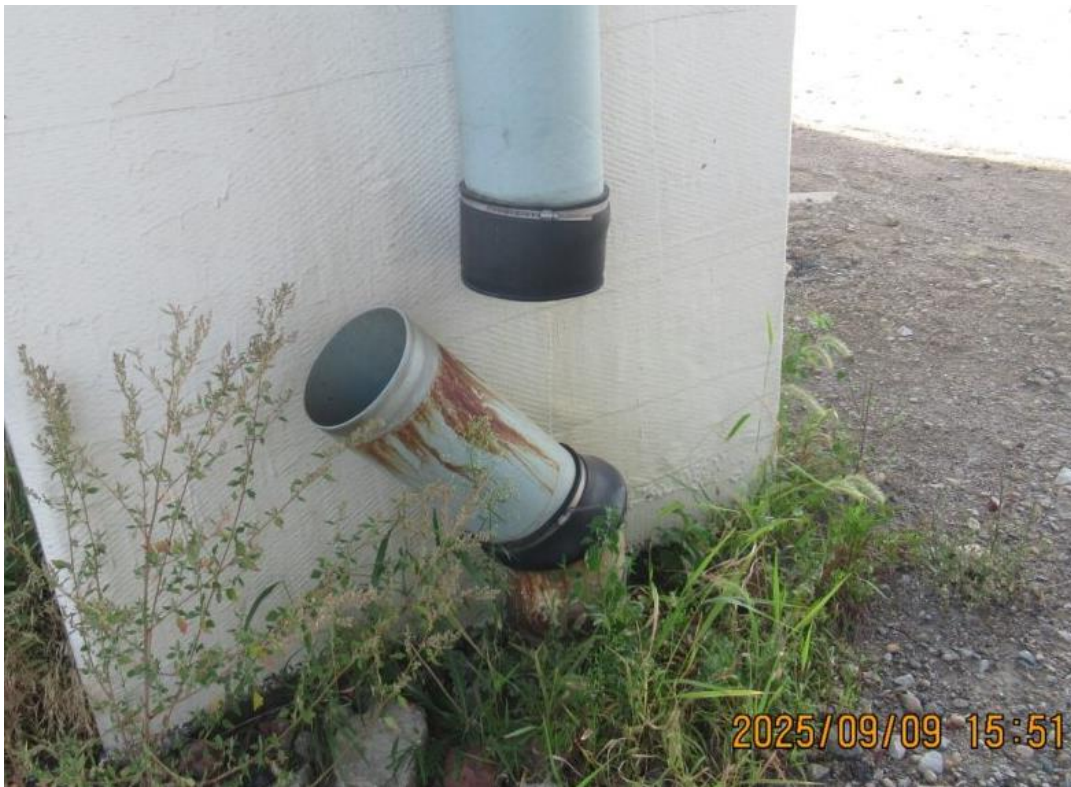
Photo 26: Disconnected drainpipe at Column 2 (Pier 19A)
