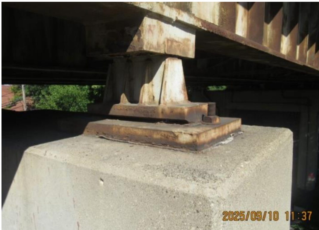
Photo 23: Pack rust under Bearing E (Pier 23A)
