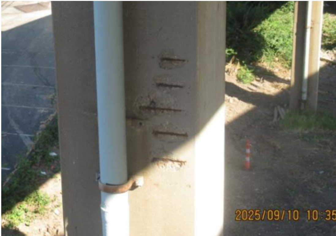
Photo 12: Multiple spalls up to 1" deep with exposed rebar on the south face of Column 1 (Pier 22A)
