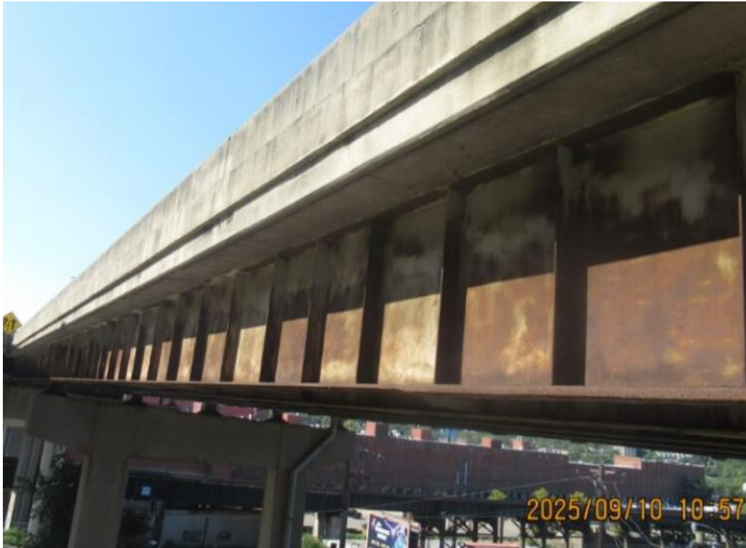
Photo 11: Typical paint condition on fascia girders (Span 22A shown)
