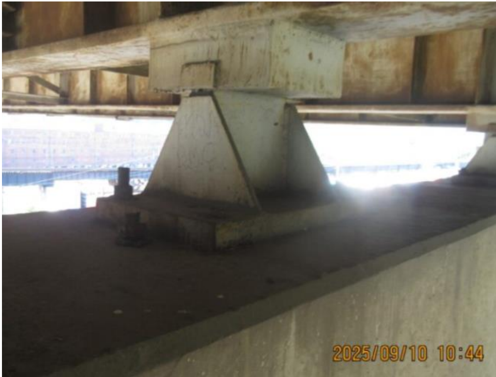
Photo 24: Broken anchor bolt (Girder C, Pier 22A)
