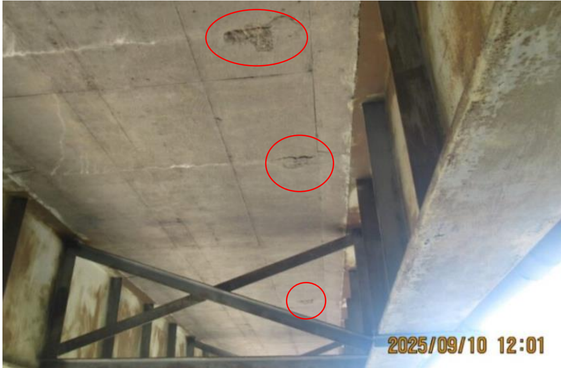
Photo 5: 3 spalls 1' dia. x 1" deep in Bay 1 (Span 24A)
