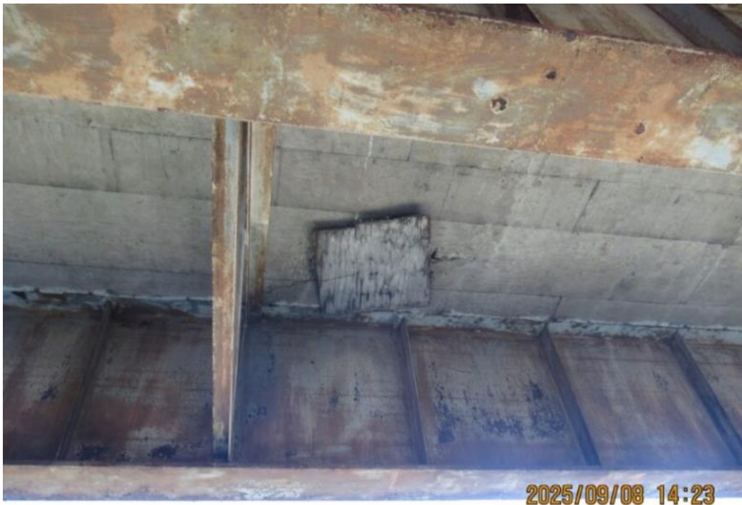
Photo 2: Typical concrete patch in deck covered with plywood in Bay 4 (Span 19C)
