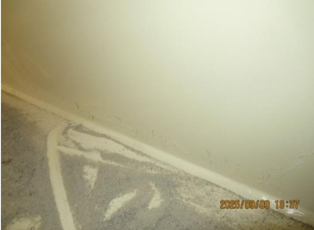
Photo 33: Typical cracking paint (Pier 25J)
