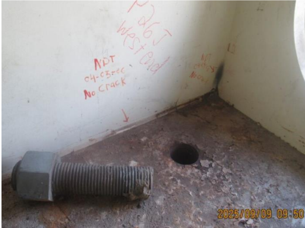
Photo 47: Broken south anchor bolt at the west column bearing (Pier 26C/J)
