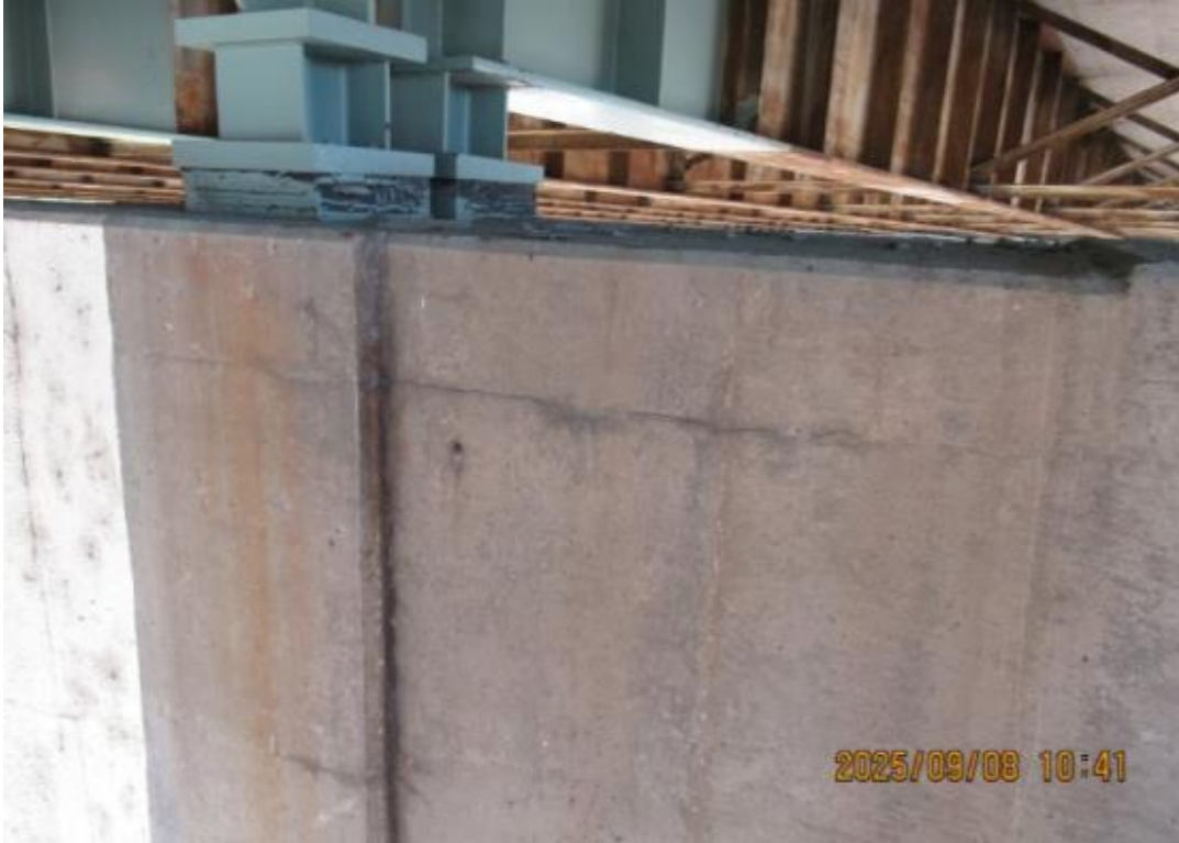
Photo 25: Typical moderate width horizontal crack near top of pier cap (Pier 15C)
