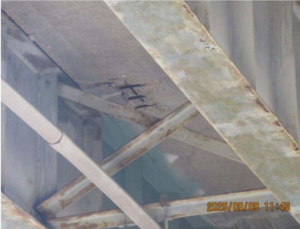
Photo 7: 3 square foot spall with exposed rebar in Bay 5 (Span 27C)
