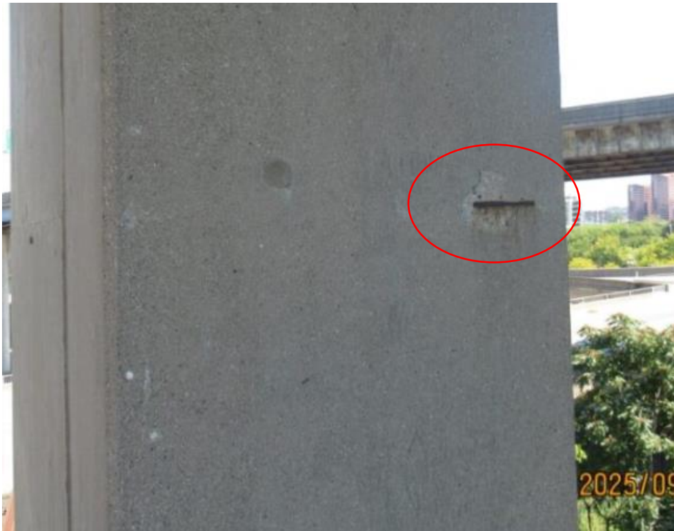
Photo 23: Exposed rebar due to shallow cover (Pier 19C)
