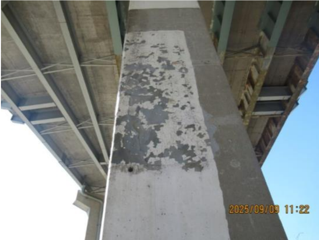
Photo 21: Cracking and peeling FRP protective coating on Column 2 (Pier 23C)
