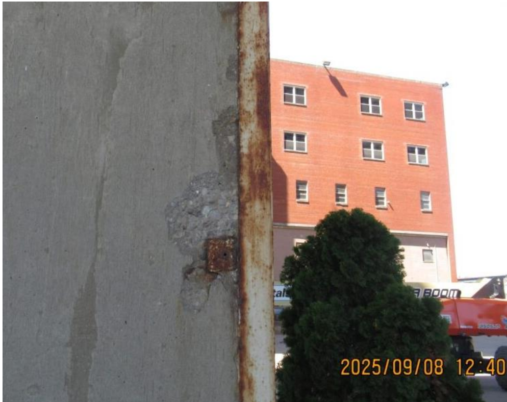
Photo 18: Typical spalling around corner armor (Pier 15C)
