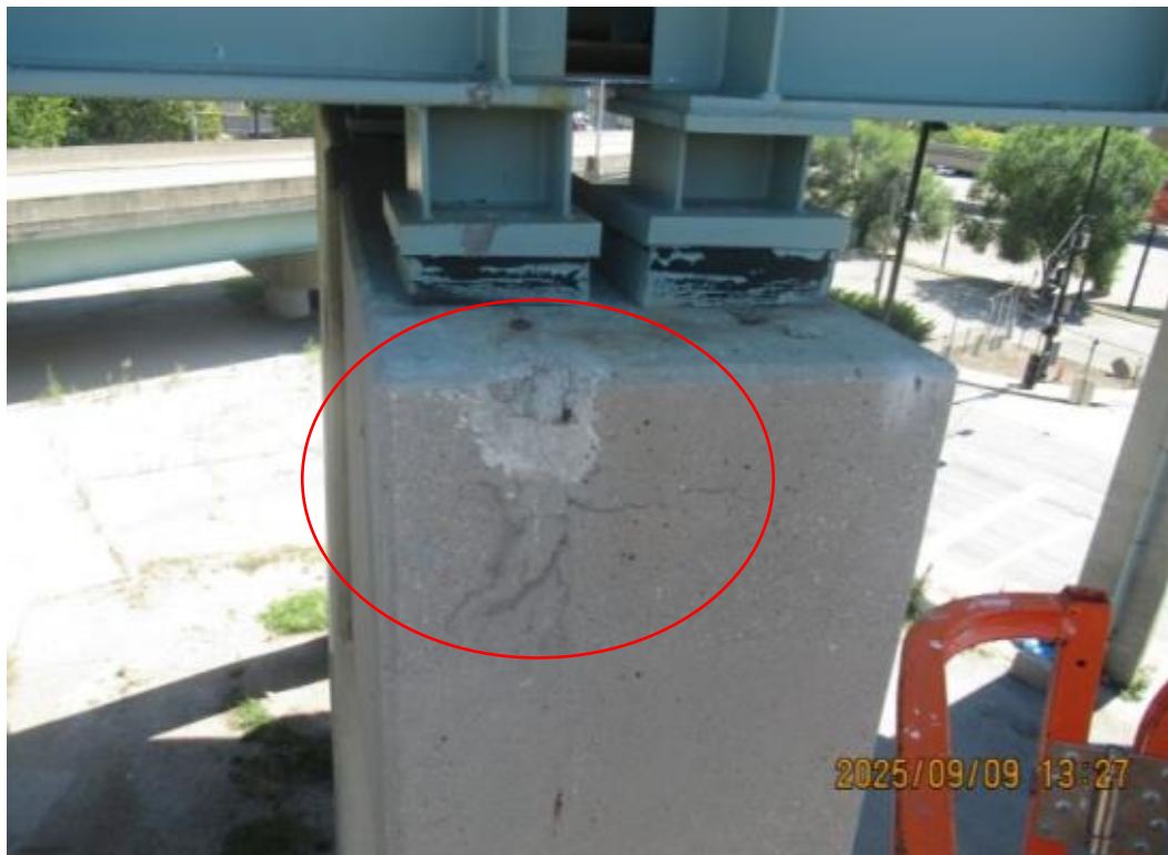
Photo 28: Map cracking with spall on west face (Pier Cap 23C)
