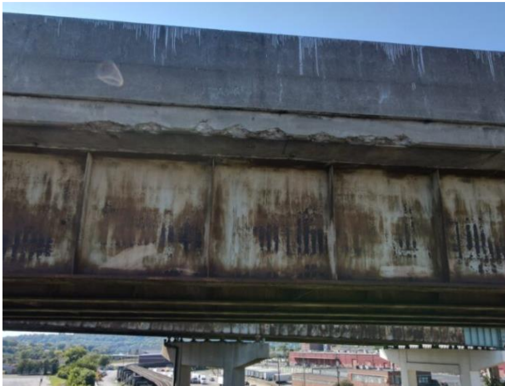
Photo 4: Continuous set of spalls up to 1" deep in the east overhang (Span 19C)
