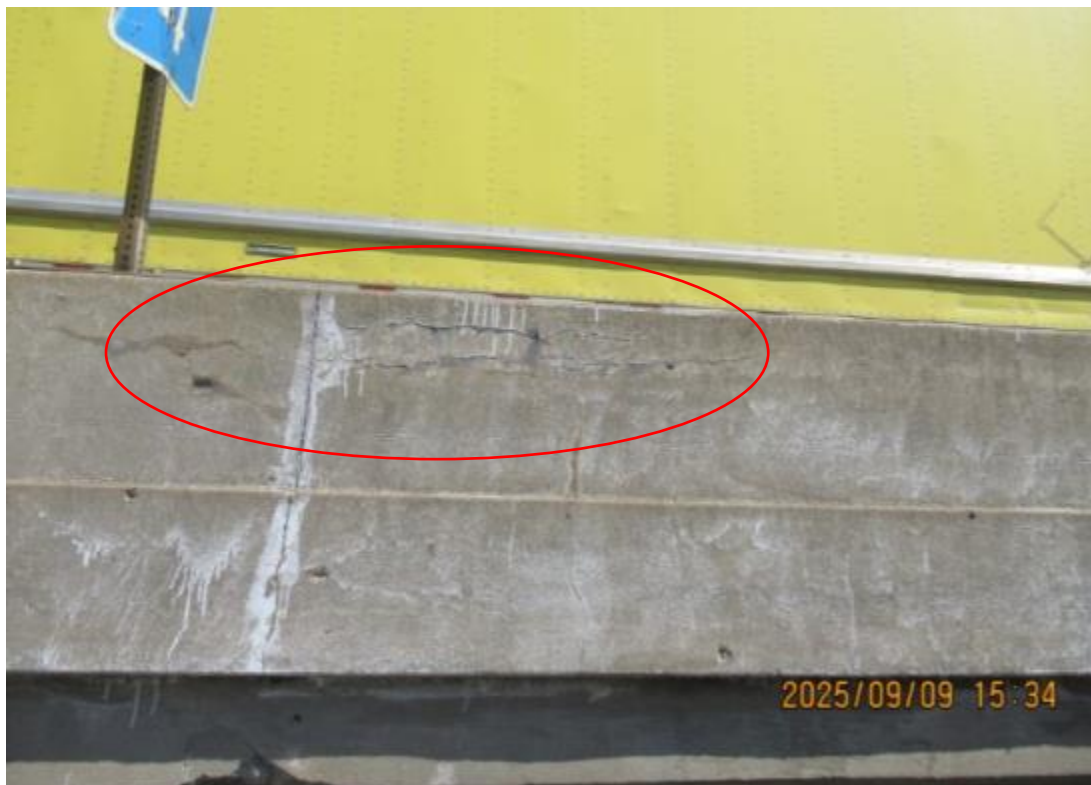
Photo 45: Map cracking in west rail above Pier 25C
