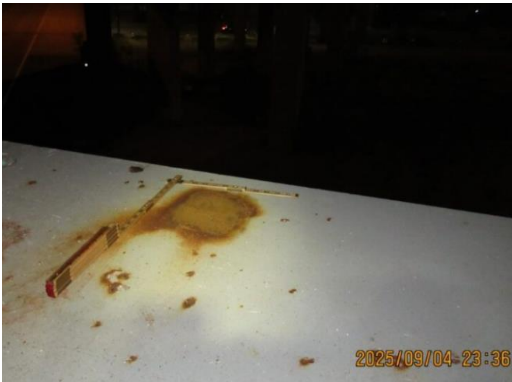
Photo 37: 6" x 6" x 3/16" deep section loss in top flange at west end (Pier Cap 26C/J)
