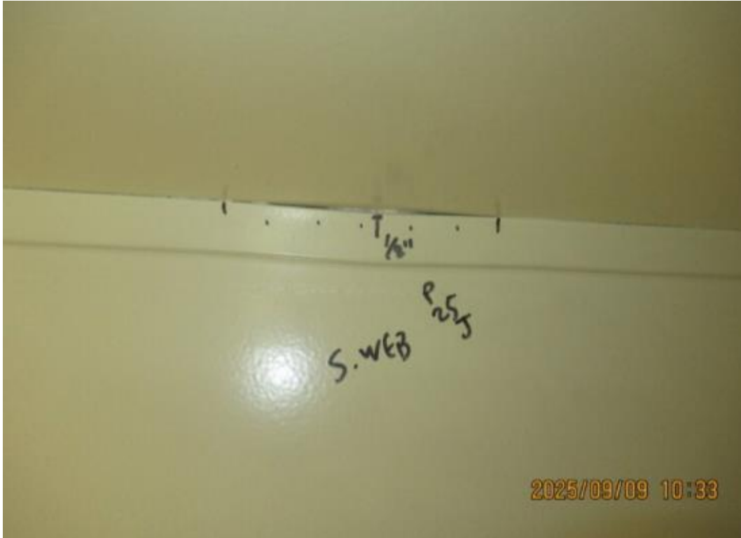
Photo 32: Top flange backer bar deflected 1/8" at east end (South Web, Pier Cap 25J)
