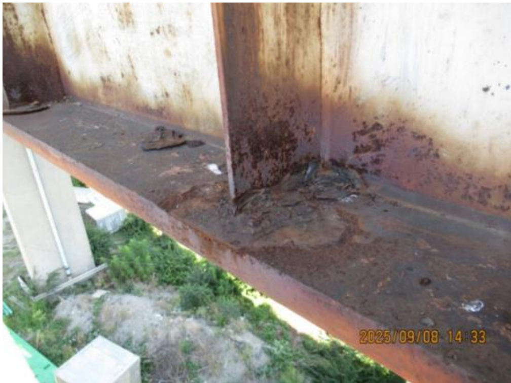
Photo 14: Laminating corrosion on bottom flange with section loss up to 9"L x 4"W x 3/16" deep (Girder A, Span 20C)
