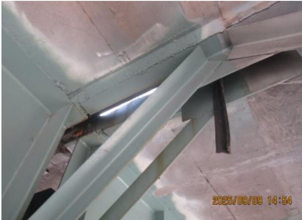
Photo 52: Failed joint seal (Pier 23C)
