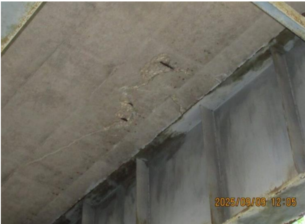
Photo 8: 2'L x 1'W x 2" deep spall with exposed rebar in Bay 5 (Span 29C)
