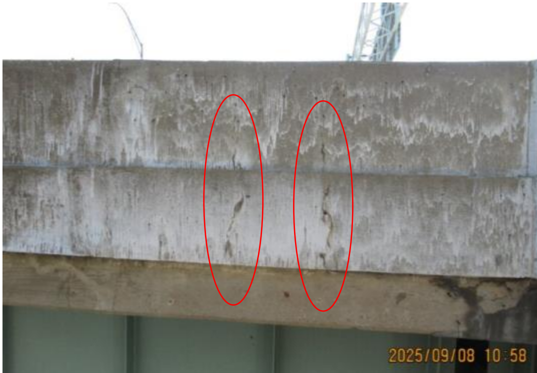
Photo 44: Typical vertical cracks in west railing (Span 16C shown)
