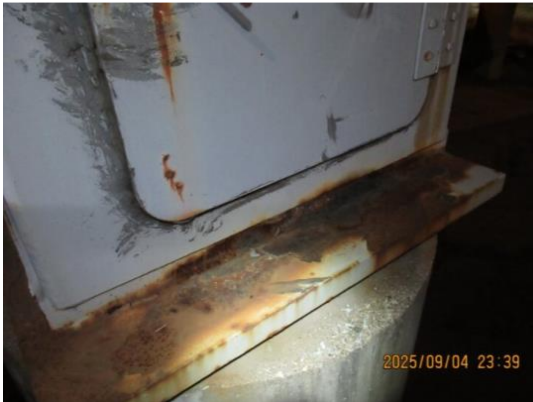
Photo 39: 1/16" deep section loss in bottom flange at west opening (Pier Cap 26C/J)
