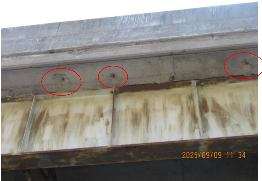
Photo 6: 3 spalls up to 1' dia. x 2" deep in west overhang (Span 26C)
