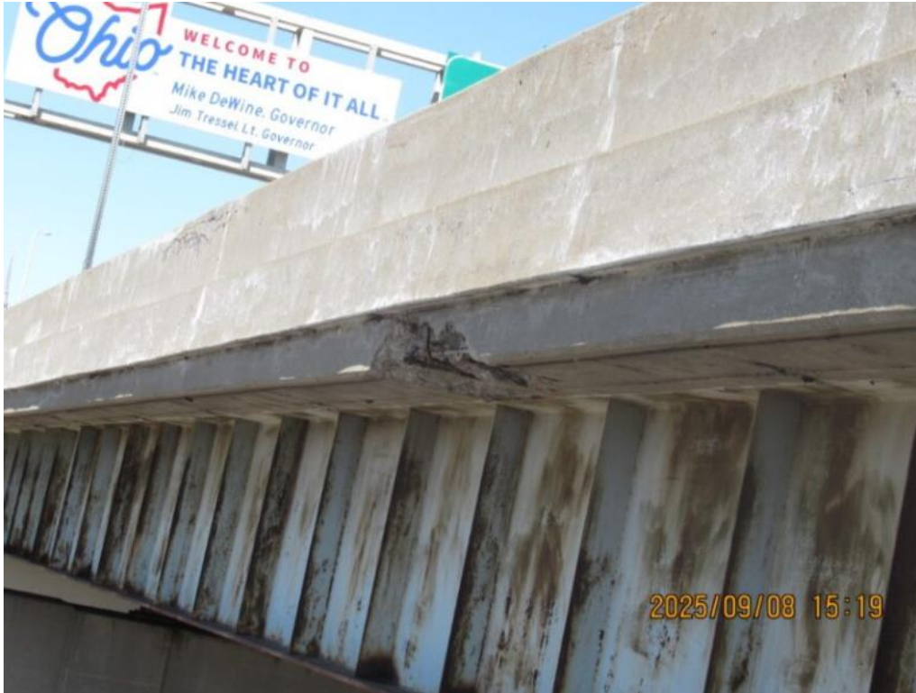
Photo 5: 3' x 2' x 4" deep spall with exposed rebar in west overhang (Span 22C)
