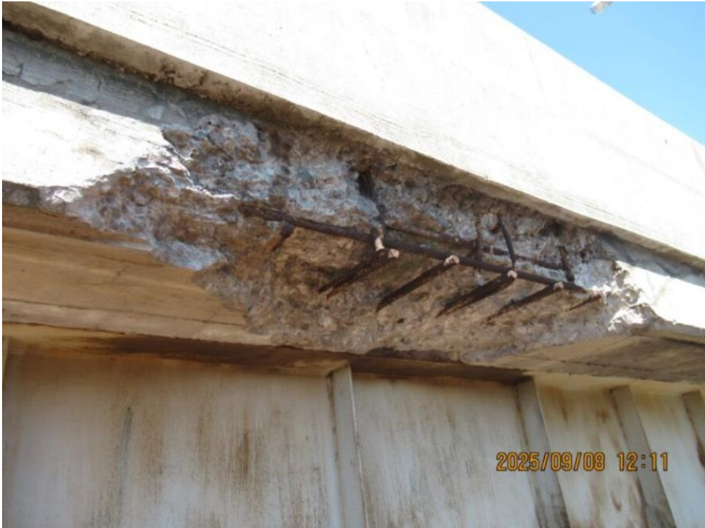
Photo 3: 6'L x 2'W x 5" deep spall with exposed rebar in east overhang (Span 17C)
