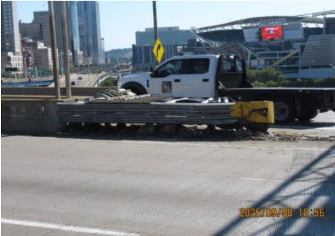
Photo 46: Impact damage to attenuator (Span 16C)
