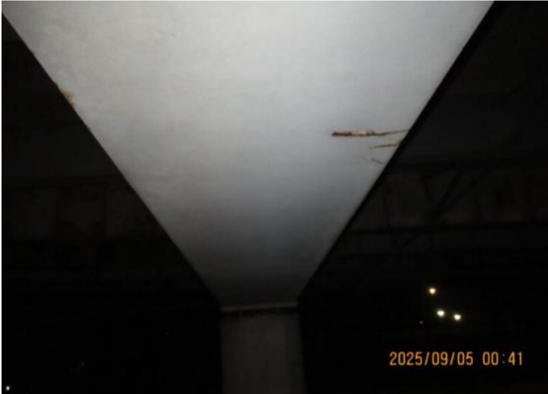
Photo 30: Scrapes with minor surface corrosion (Pier Cap 25J)
