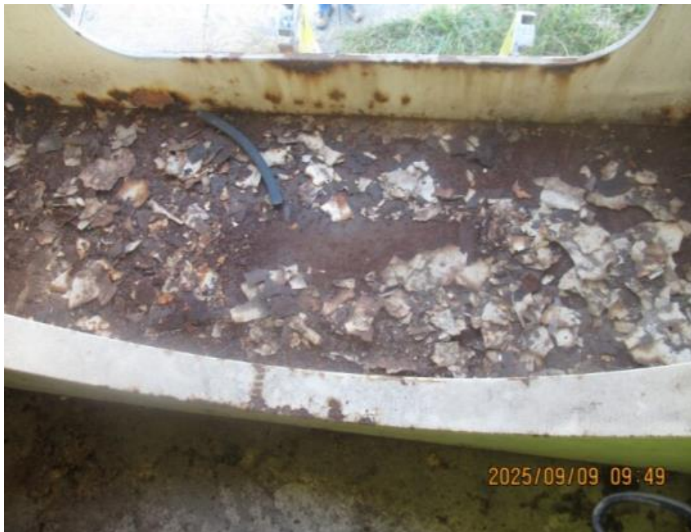
Photo 40: Surface corrosion with pitting less than 1/16" deep at west end (Pier Cap 26C/J)
