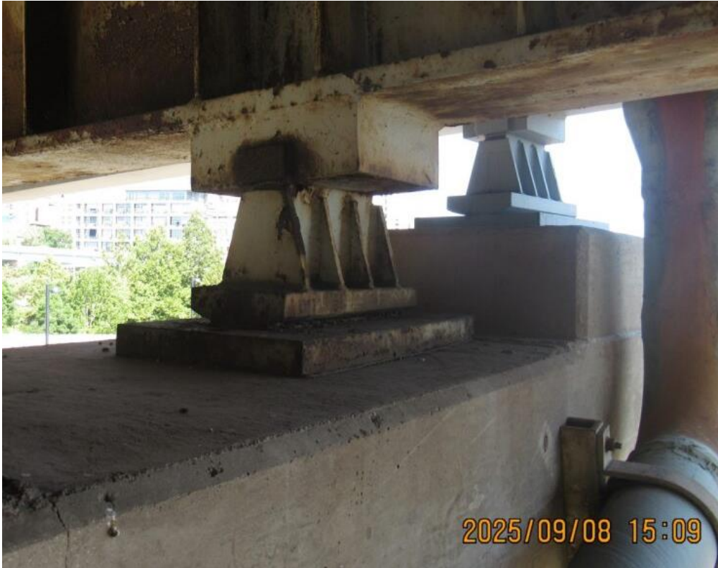
Photo 48: Pack rust under Bearing E (Pier 21C)
