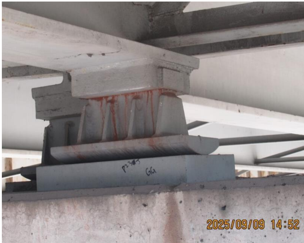
Photo 49: Minor fretting corrosion on Bearing G (Pier 23J)
