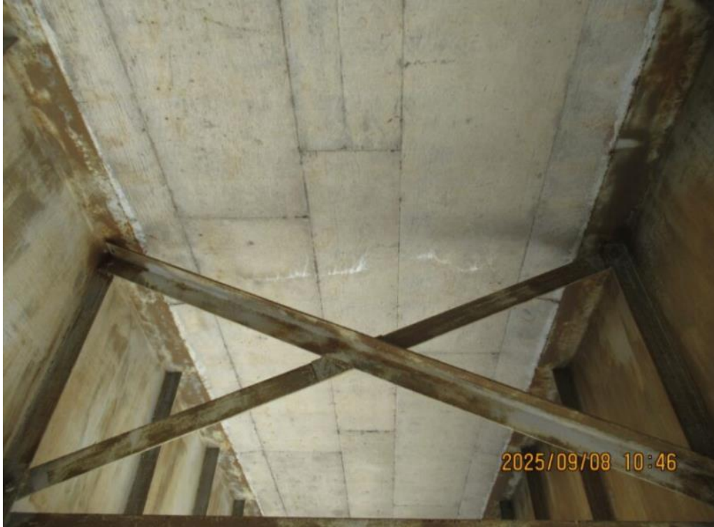
Photo 1: Typical transverse crack with efflorescence (Span 16C shown)
