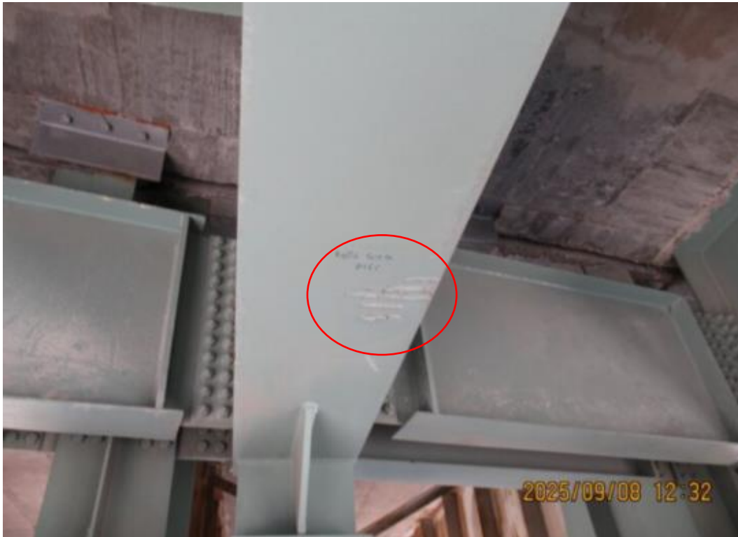
Photo 16: Gouges up to 5" long and 1/8" deep on bottom flange (Girder D, Span 16C)
