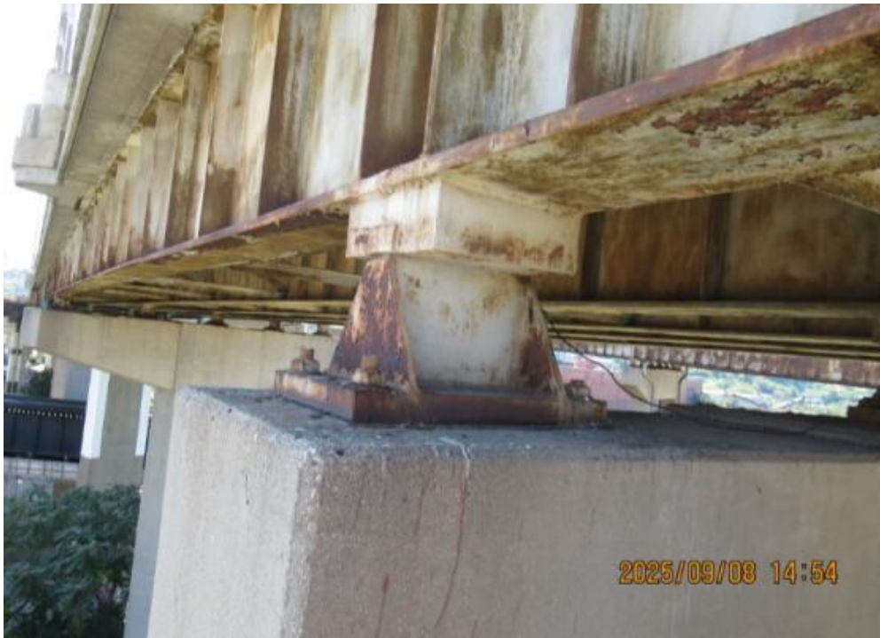
Photo 51: Typical surface corrosion on fascia bearing (Pier 20C)
