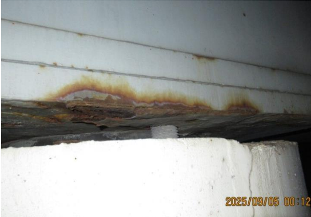
Photo 38: Laminating corrosion on bearing plate at Column 2 (Pier Cap 26C/J)
