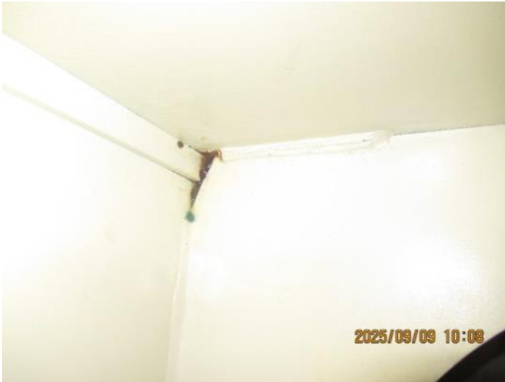
Photo 42: Minor surface corrosion at top corners of Diaphragm 17 sealed with silicone (Pier Cap 26C/J)
