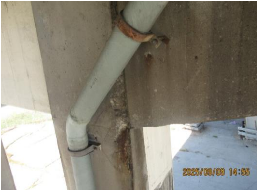
Photo 20: 4'H x 1'W x 2" deep spall with exposed rebar and delamination on Column 2 (Pier 23C)
