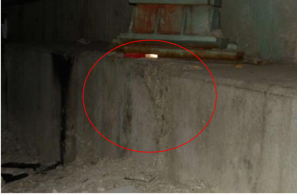
Photo 24: Spall and delamination below Bearing E (Abutment C)
