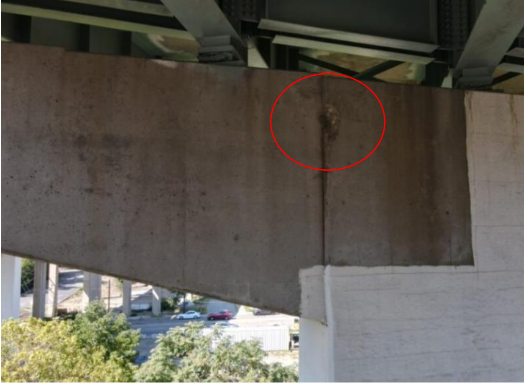
Photo 27: 16"H x 6"W x 1 1/2" deep spall on the south face (Pier Cap 18C)
