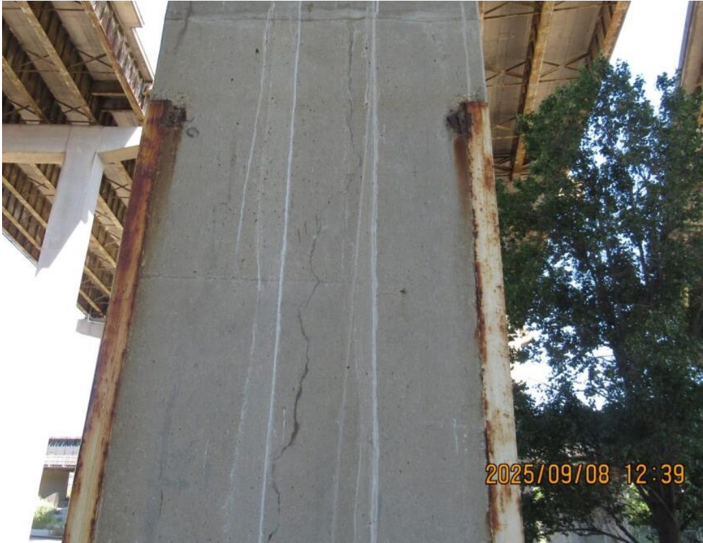
Photo 19: Moderate-width vertical crack on Column 1 (Pier 15C)
