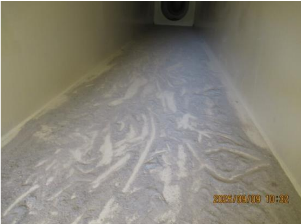
Photo 34: Debris inside pier cap (Pier Cap 25J)
