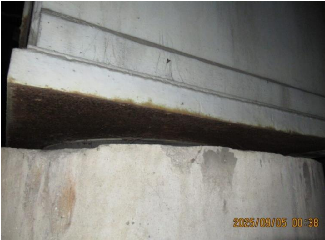
Photo 31: Surface corrosion on the underside of the west bearing (east bearing similar, Pier Cap 25J)
