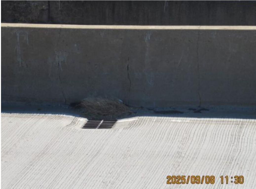
Photo 53: Vegetation/debris accumulation in a scupper (Span 16C)
