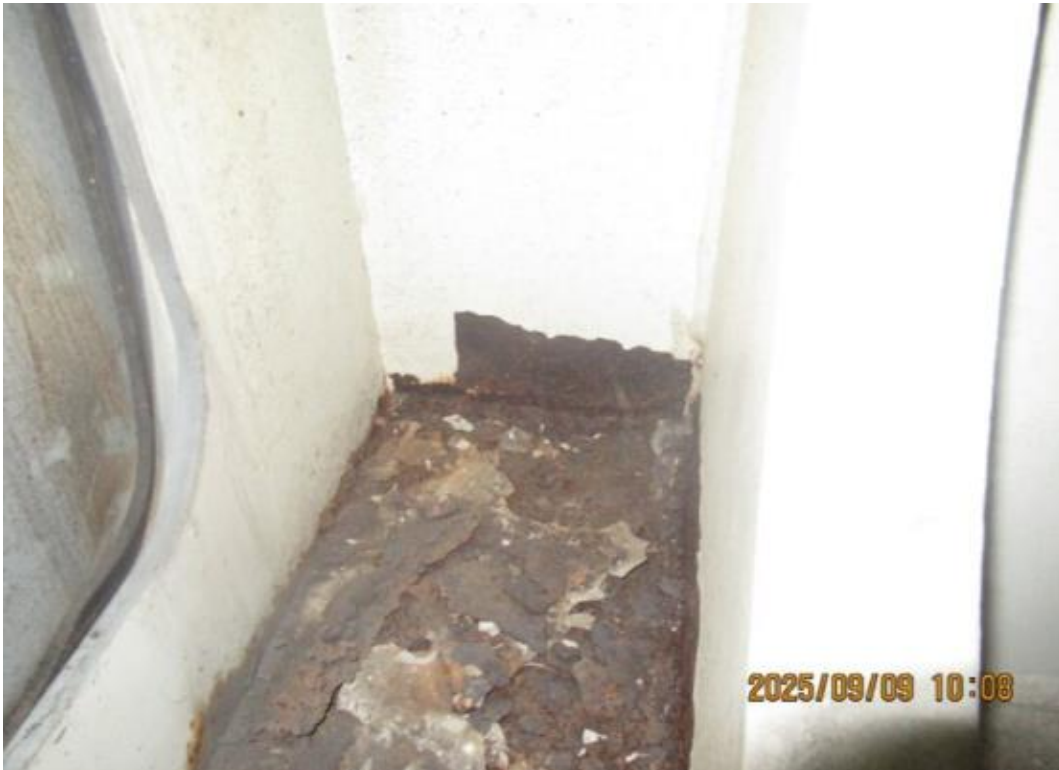
Photo 41: Laminating corrosion with section loss up to 1/8" deep at east end (Pier Cap 26C/J)
