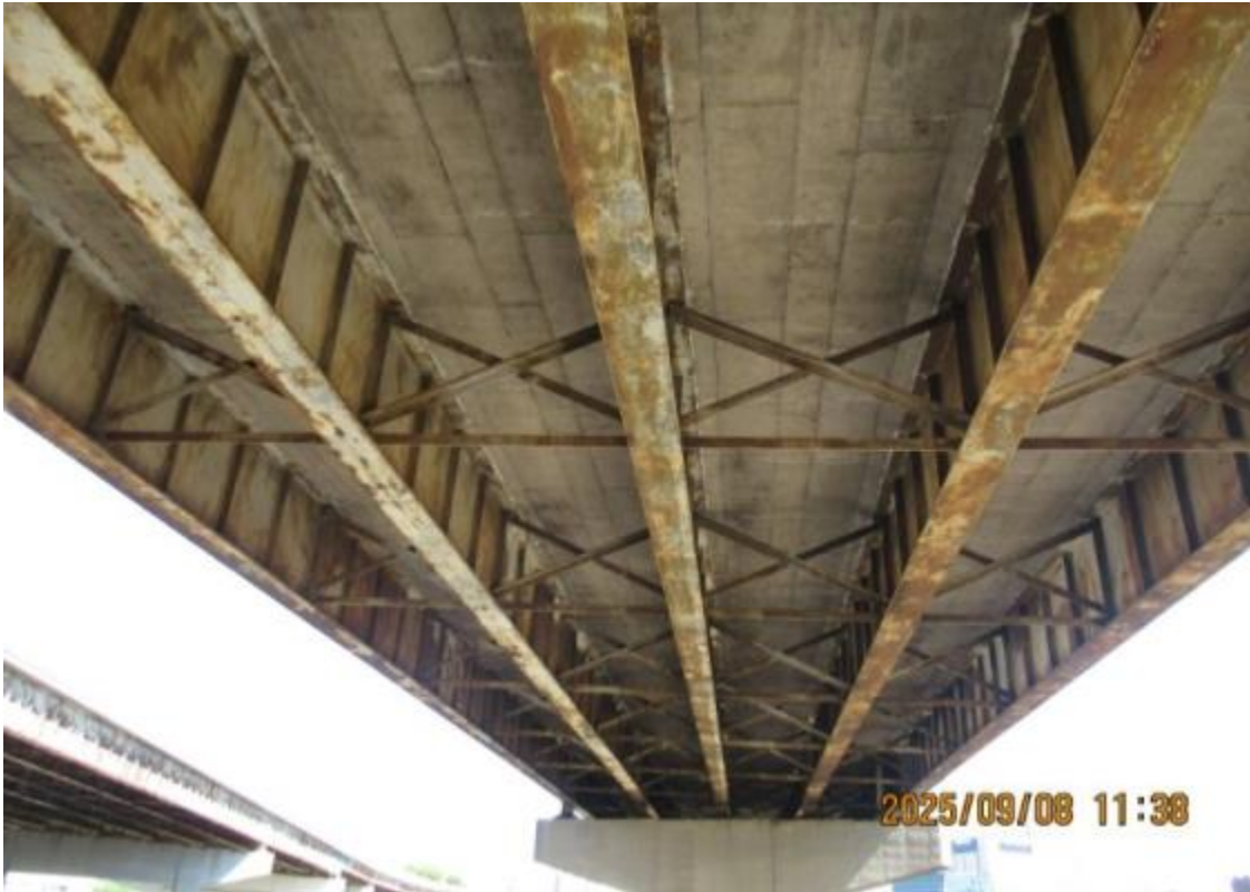
Photo 17: Typical original girder paint condition (Span 17C shown)
