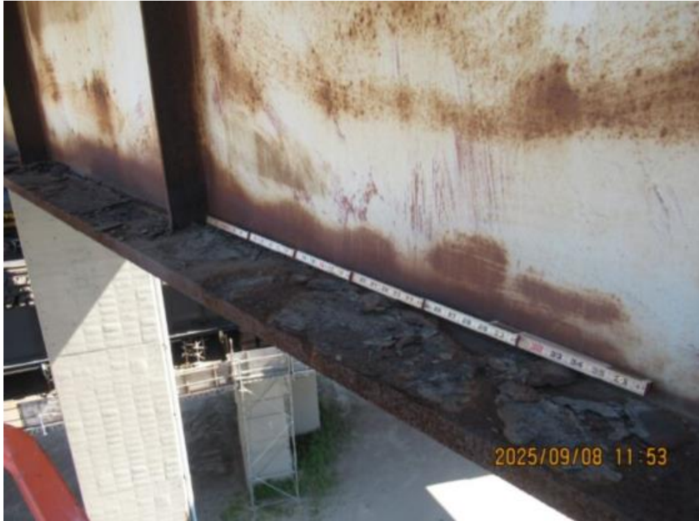
Photo 15: Laminating corrosion with section loss up to 8"W x 1/4" deep near midspan (Girder A, Span 17C)
