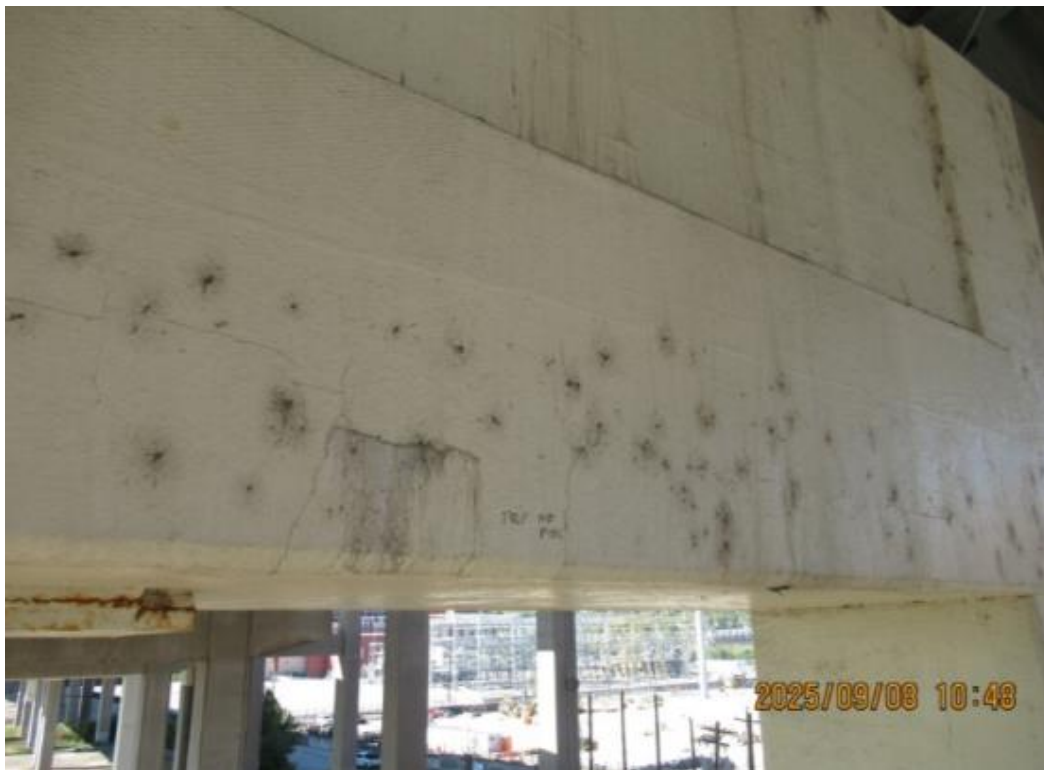
Photo 26: Moderate width vertical cracks and map cracking (Pier 15C)
