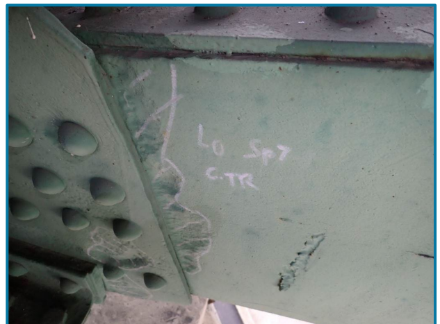
Photo 39 – 3/16" deep section loss to the lower chord adjacent to the gusset plate (L0L1 of the Center Truss, Span 7).
