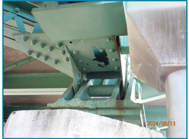
Photo 41 – 10" H x 6" W corrosion hole in the lower batten plate at the bearing (L0 of the North Truss, Span 5).
