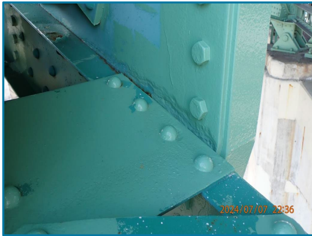
Photo 73 – 3/16" painted over pitting adjacent to the lower chord (L1, North Truss, Span 10).
