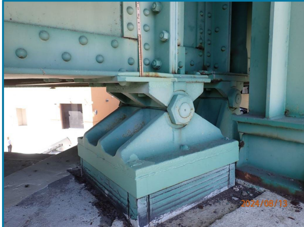
Photo 75 – 3/16" pack rust between the lower chord and the bearing (North Truss, Span 4, looking southwest).
