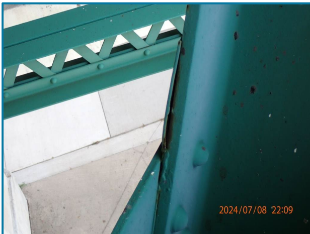
Photo 59 – 1/8" pack rust at the fill plate causing distortion to the plate (U16L17 of the North Truss, Span 8).
