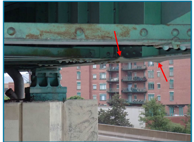
Photo 27 – Bent bottom flange (Span 12 shown, looking southeast).
