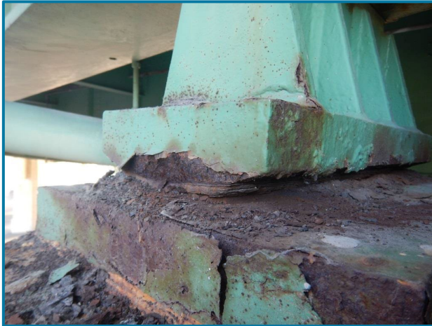
Photo 9 – 1/2" pack rust between the rocker and the masonry plate (Girder A, Pier 2, Span 3, looking south).
