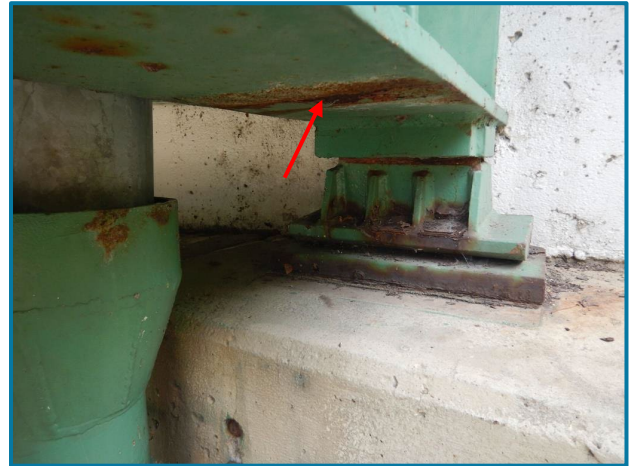
Photo 7 – Surface corrosion to the girder bottom flange (Girder A, Span 1, looking north).
