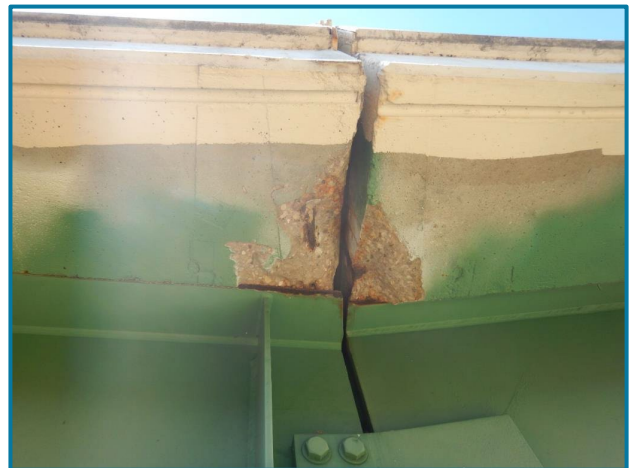
Photo 3 – 1'-6" L x 1' W x 6" D spall in the deck overhang (Girder A, Spans 1-2, looking west).
