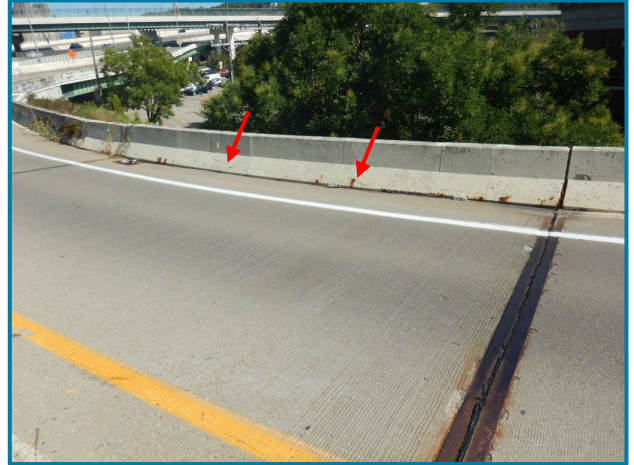
Photo 5 – Bridge railing with longitudinal cracking with rust stains (looking east).
