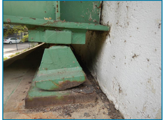
Photo 10 – Corrosion to the bearing and Girder A contacting the backwall (Girder A, Rear Abutment, 4, looking west).
