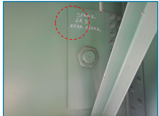
Photo 8 – Gouges in the plate at the hinge over Pier 1 (Pier 1, Girder A, looking east). The markings on the bridge as shown in the photo are incorrect.
