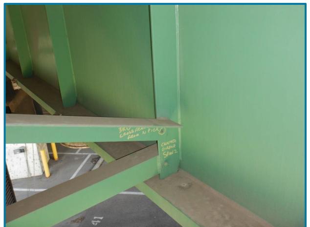
Photo 12 – Insufficient weld length and missing connection (Girder A, Span 2, looking north).
