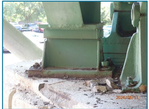
Photo 11 – Loose anchor nut and section loss (Girder A, Pier 4 (HAM-50-2180N), Span 3, looking east).
