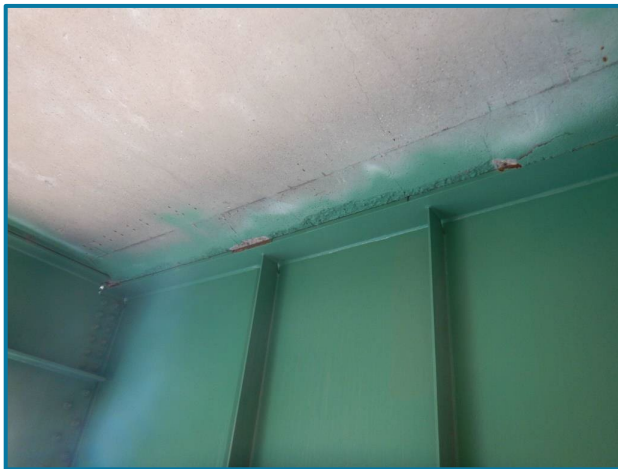
Photo 2 – 8' L shallow haunch spall in the deck (Girder A, Span 2, looking northeast).
