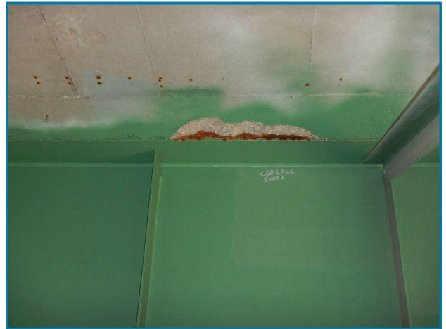
Photo 1 – 2' L haunch spall in the deck (Girder B, Span 2, looking southwest).
