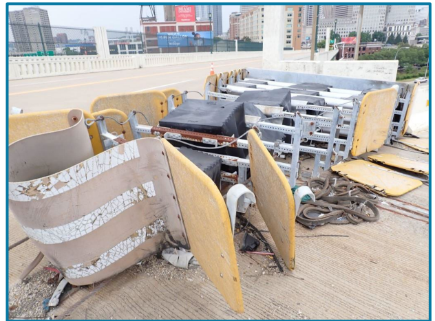
Photo 13 – Impact damage to the crash attenuator at the exit (South Approach, looking west).
