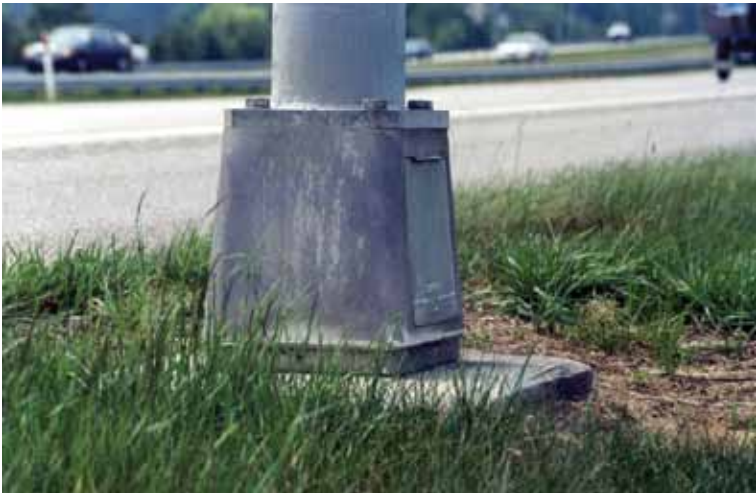
Figure 4-11. Example of a Cast Aluminum Frangible Luminaire
