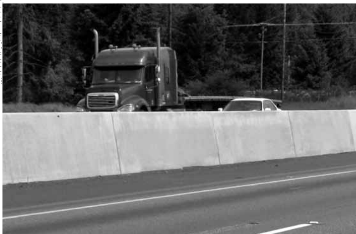
Figure 5-20. Constant Slope Barrier
