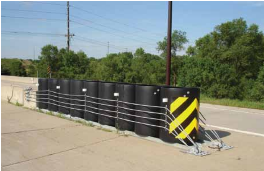
Figure 8-36. Reusable Energy-Absorbing Crash Terminal (REACT 350®)
