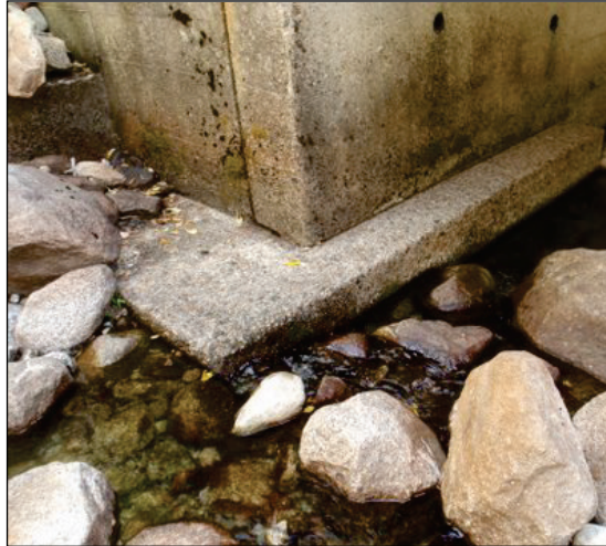
Figure 6.9. Exposed spread footing in an open-bottom culvert.
