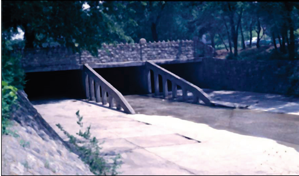
Figure 2.8. Concrete debris fins with sloping leading edge as extension of culvert walls.
