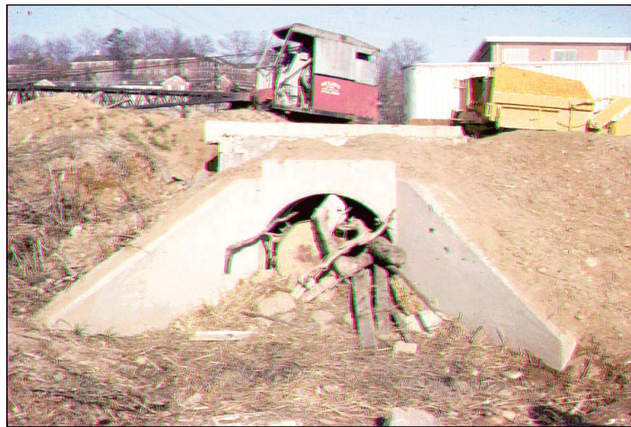
Figure 6.3. Severe debris blockage.
