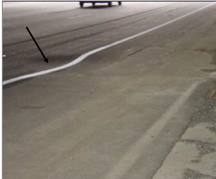
Figure 6.2. Roadway settlement caused by voids around a culvert.
