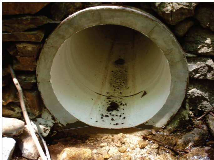
Figure 6.12. Slip lining a 30 inch (750 mm) CMP with a 24 inch (600 mm) PVC pipe.
