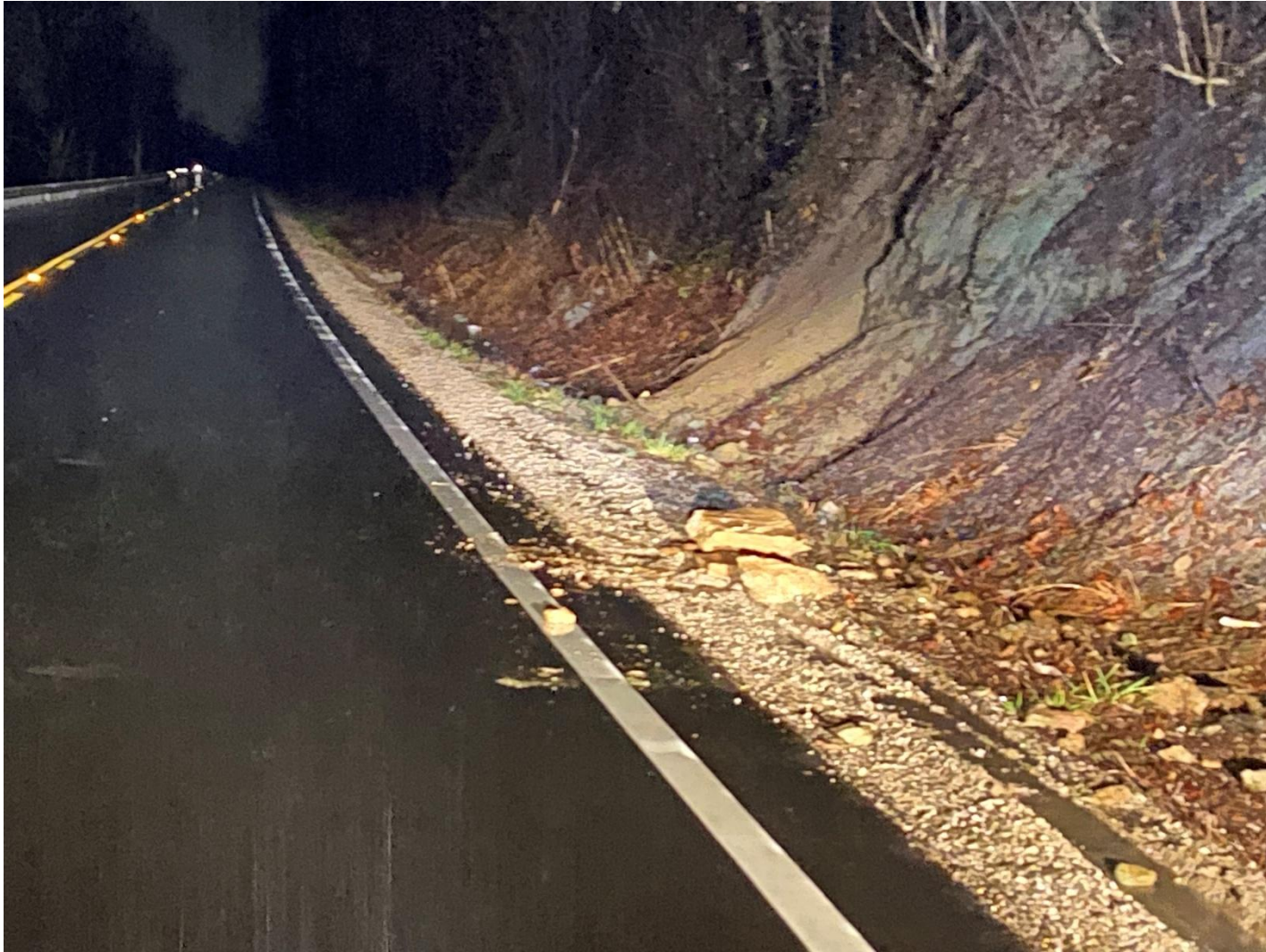
Photograph 1: Rockfall at about MM 17.415 impacting the edge of roadway during the night of January 31, 2025.
