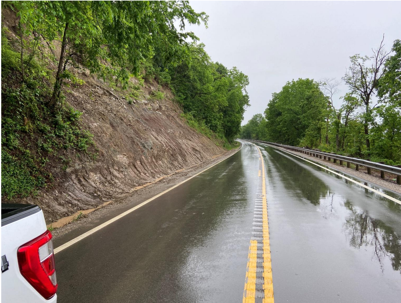
Photograph 8: Areas where debris/rock was removed from ditches at about MM 17.43 in May 2025. Note, the County removed debris fall is ditches over nine days during the month of May in the following approximate MMs: 17.43, 17.9, 18.1, 18.5, and 19.03.
