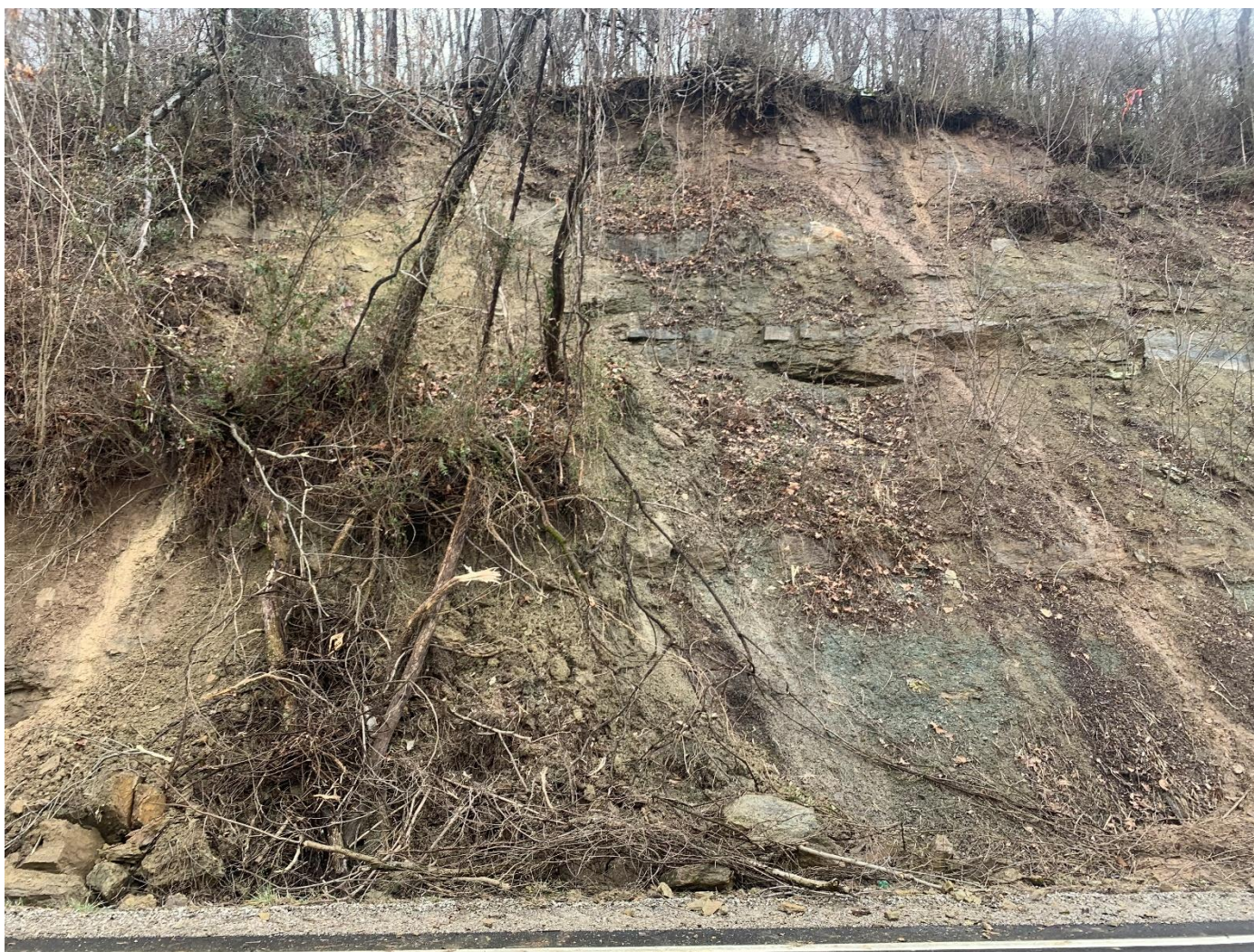
Photograph 2: Debris and fallen trees impacting the shoulder at MM 17.415 on February 6, 2025.
