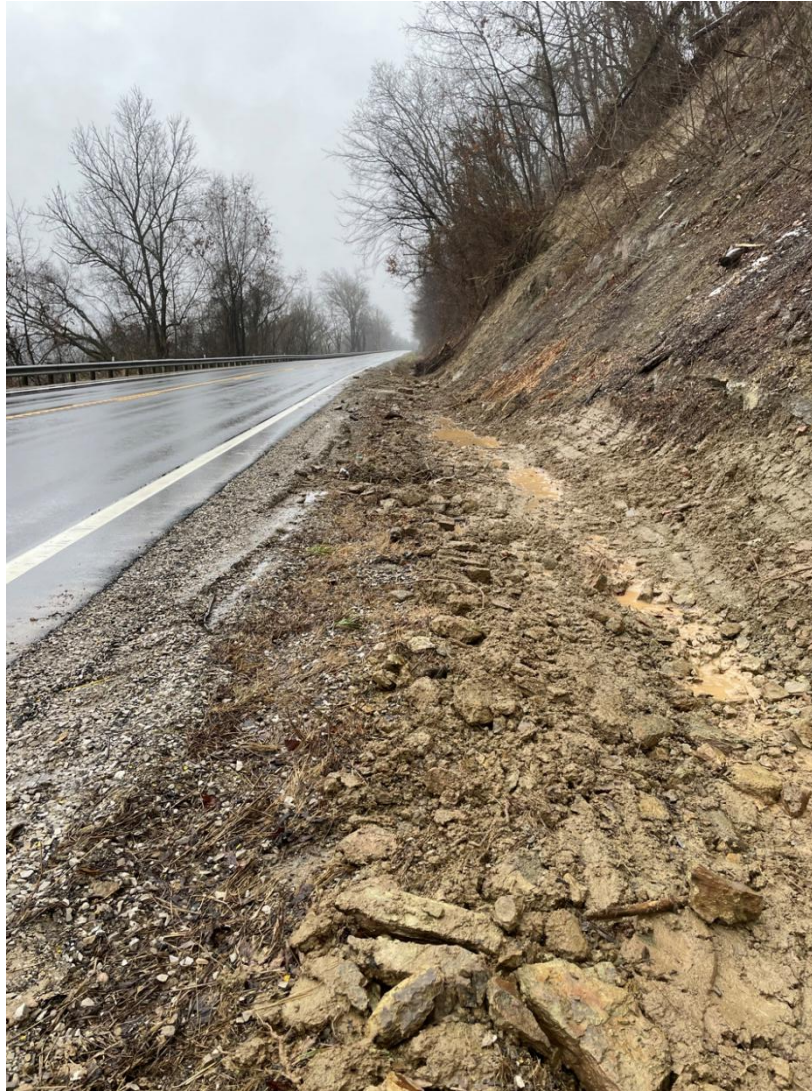
Photograph 7: Historical photograph from rockfall accumulation in the ditch near to MM 17.44.
