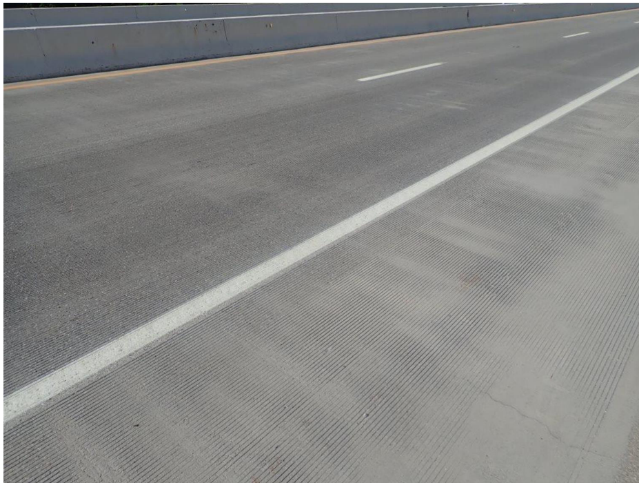
PHOTO 19 Description Typical view of the deck, southbound lanes of Span 3 shown (looking southeast)
