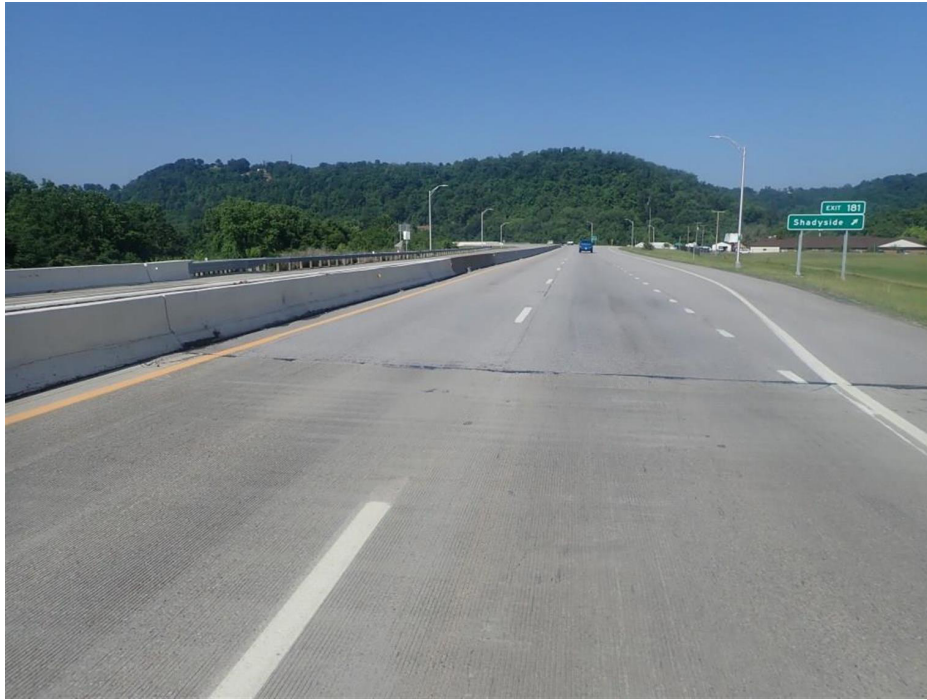
PHOTO 1 Condition Description Rear approach roadway looking away from the bridge, southbound lanes shown (looking south)
