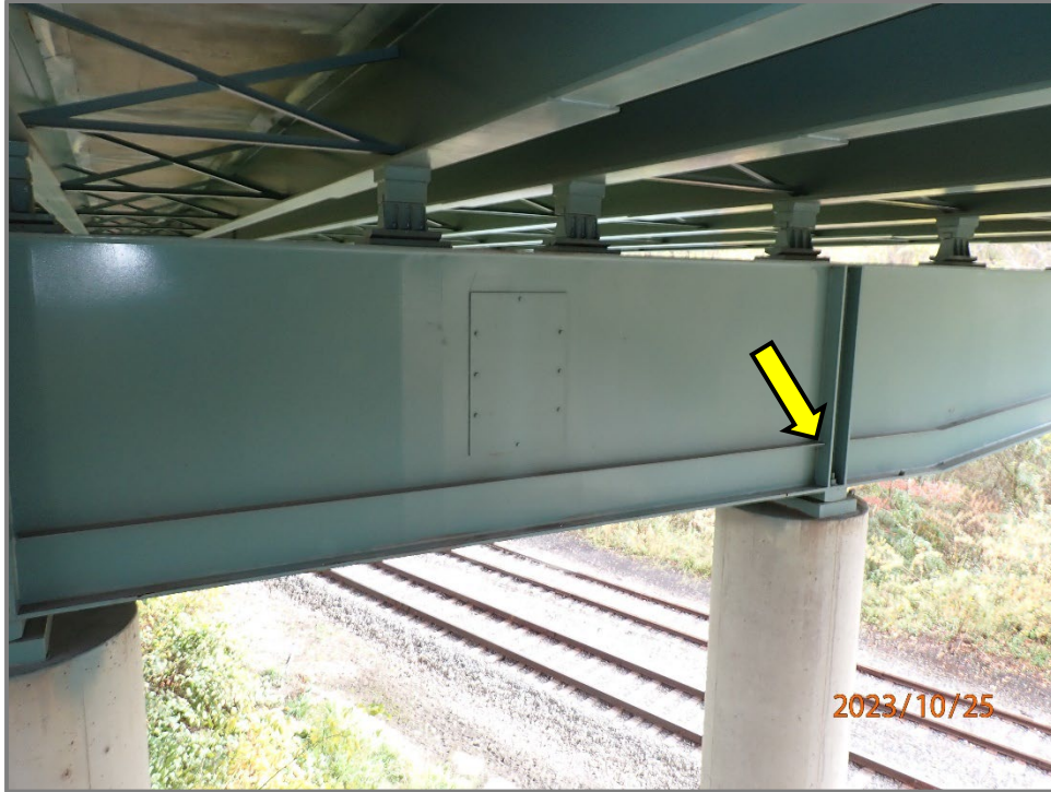
Photo 1 – Base metal at the end termination of longitudinal stiffener to girder web welds with no transition radius (Category E). South face of the Pier 1 cap shown, looking north.
