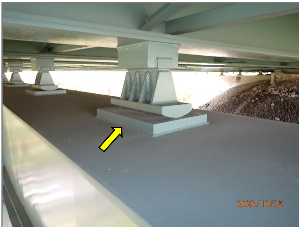
Photo 2 – Base metal at bearing sole plate to top flange longitudinal welds ( t \geq 1'' ) (Category E'). Girder 2 bearing at Pier 1 cap shown, looking southeast.
