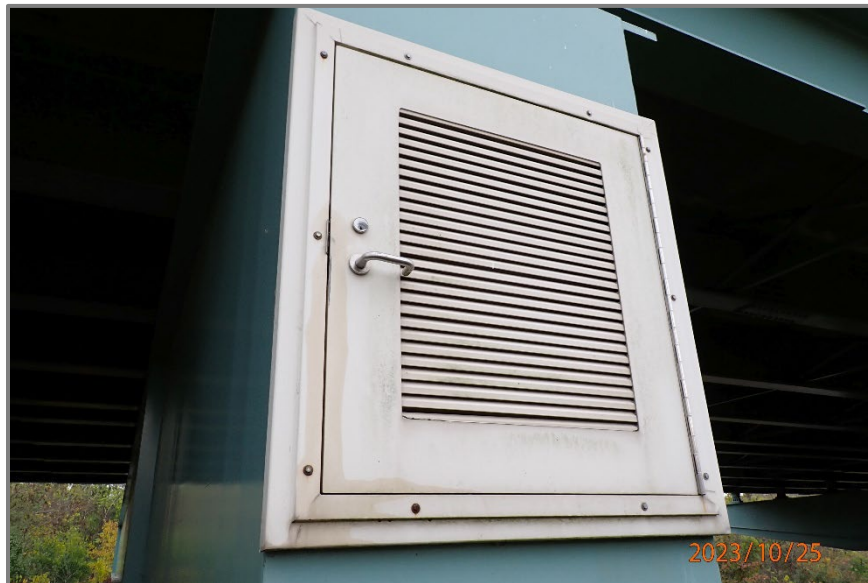
Figure 6 – Typical access door on end of cap, looking east at the west end of the Pier 2 cap.
