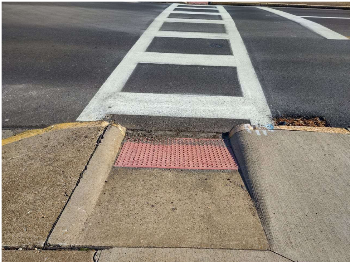
Photo 4: Sunken curb ramp creating a hazard for pedestrians, especially those in wheelchairs. Source: OMEGA
