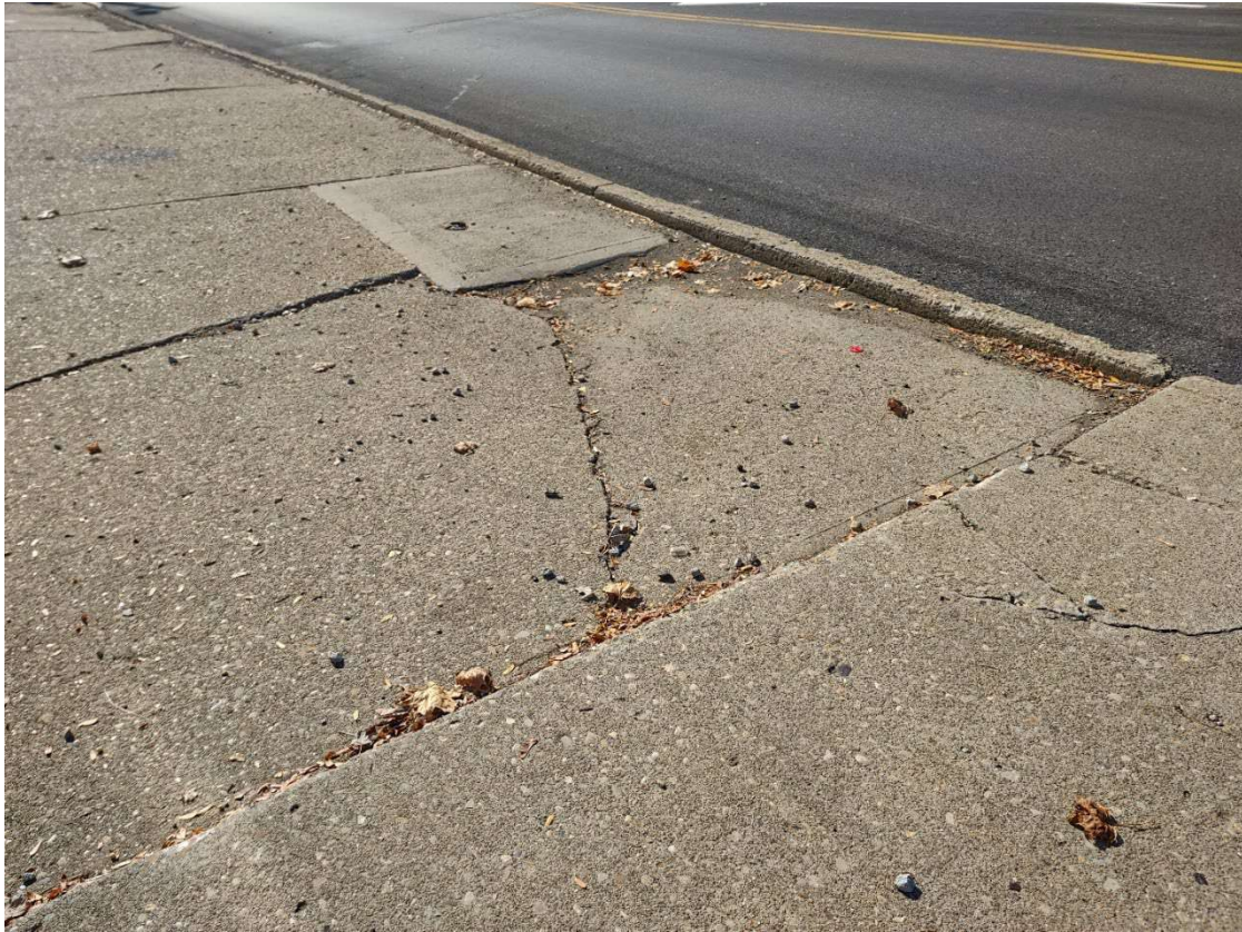
Photo 5: Cracked and sunken sidewalk creating a roughly 3 inch tripping hazard. Source: OMEGA
