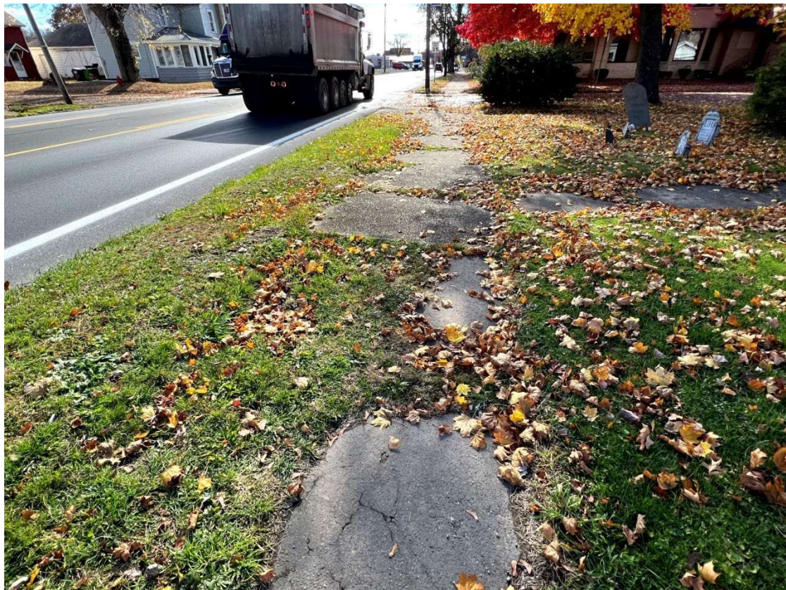
Photo 6: Cracked/missing Sidewalk that has since been overgrown. Source: OMEGA
