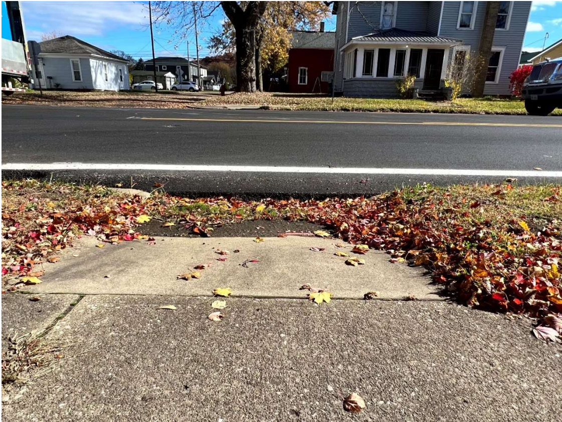
Photo 3: ADA ramps need rebuilt and leveled to new surface of the road. Source: OMEGA.
