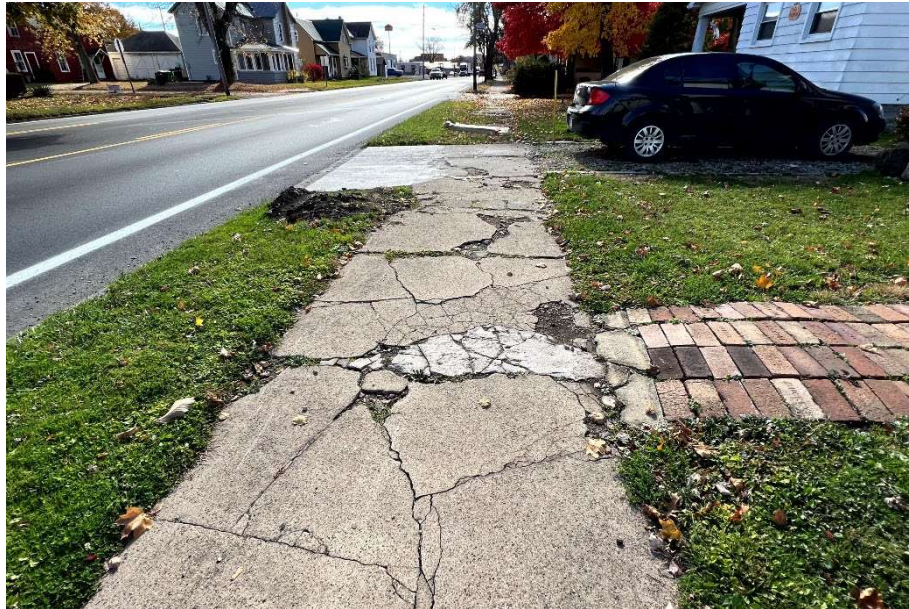
Photo 1: Cracked and uneven surfaces, indicative of many sidewalks along Wooster Avenue. Source: OMEGA
