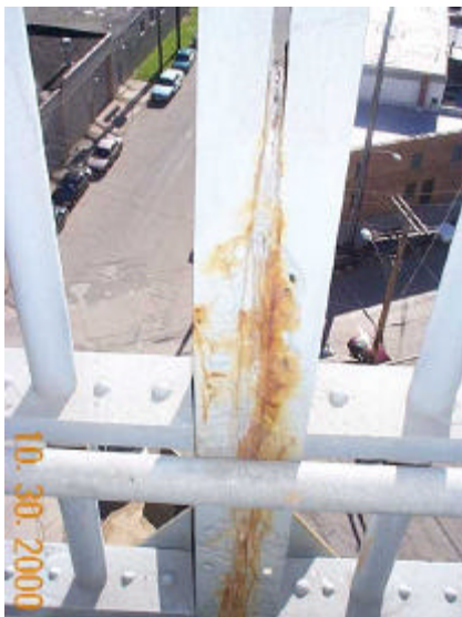
Photo 12 – Packrust to main span exterior railing posts dcp00071.jpg
