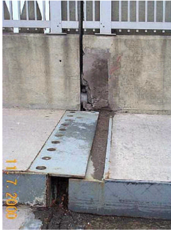
Photo 5 – Spalled patch to north rail at panel point 0'
