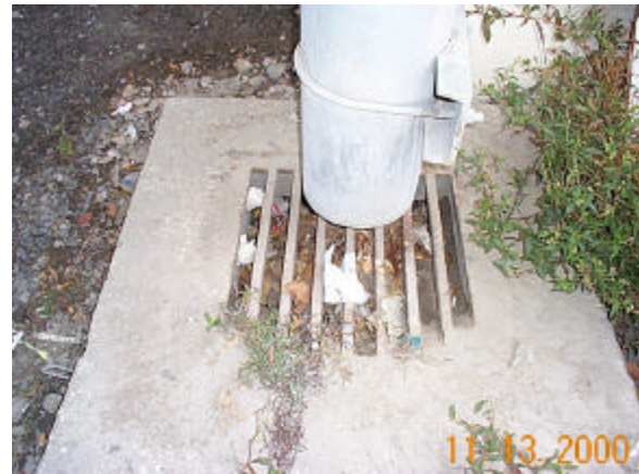
Photo 18 – Pier 9 South Exterior clogged
