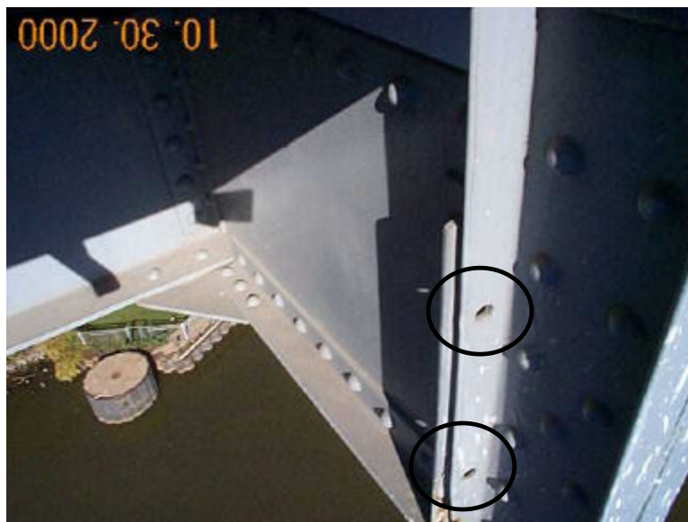
Photo 16 – Missing bolts between lower deck floorbeam and railing dcp00072.jpg
