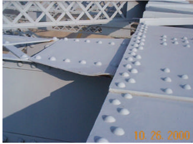
Photo 59 - Bent Gusset at U5', South Arch
