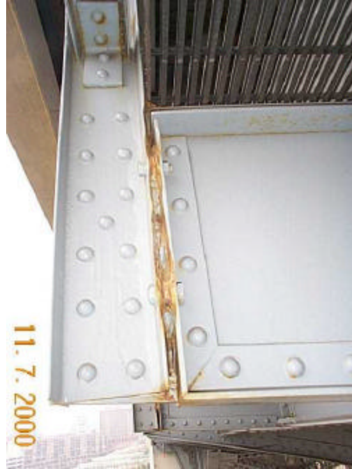
Photo 15 – Packrust between lower deck floorbeam and railing dcp00195.jpg
