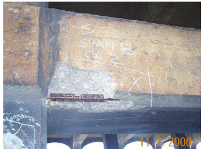
Photo 9 – Spall with exposed reinforcing to center bay railing dcp00112.jpg
