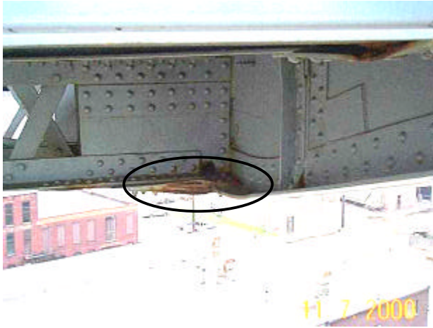
Photo 58 - Packrust at 8', South Arch
