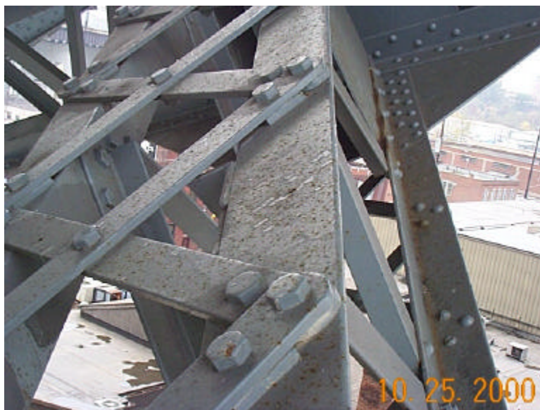
Photo 44 – Debris under paint
