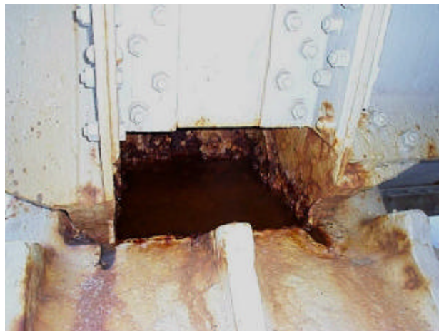
Photo 60 - Standing water at L0', North Bearing
