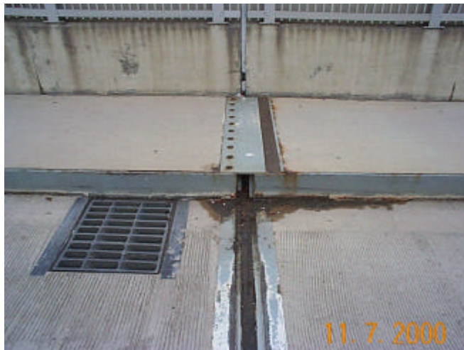
Photo 19 – Debris Accumulation at Gutter at Expansion Joint dcp00186.jpg
