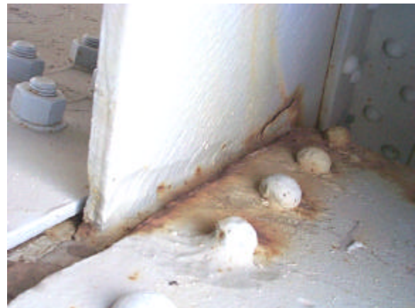
Photo 50b - North Arch South Gusset Plate at L1' dcp00330.jpg
