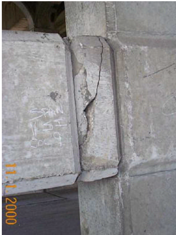
Photo 8 – Crack to center bay railing dcp00111.jpg
