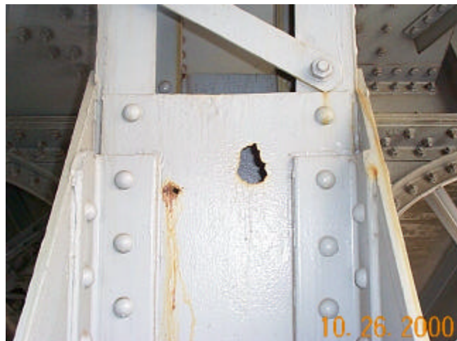
Photo 50 - South Arch Diagonal U3-L4
