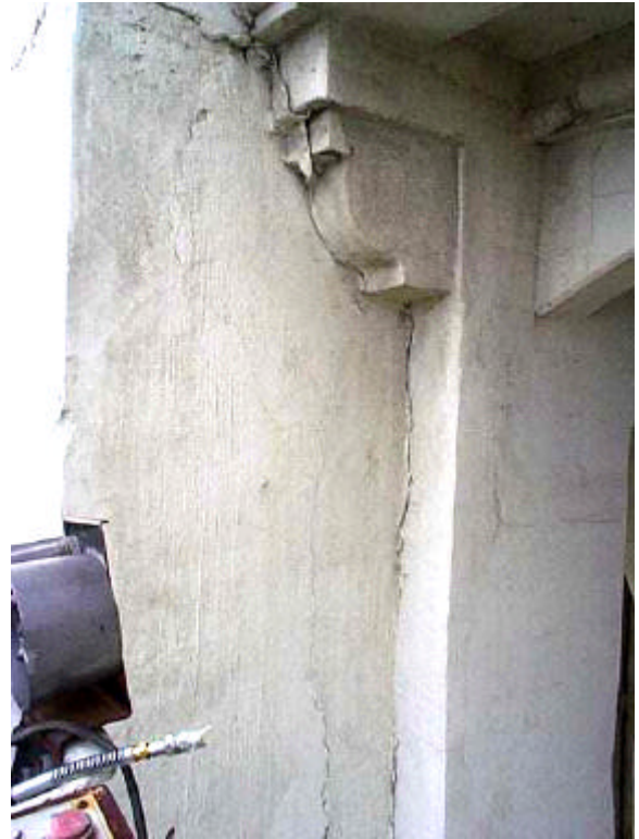
Photo 2 - Pier 6, Southeast corner delamination and spall forming
