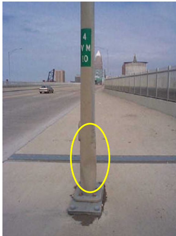
Photo 5 - Impact damage to light post 4 VM 10 at the South sidewalk of the West approach
