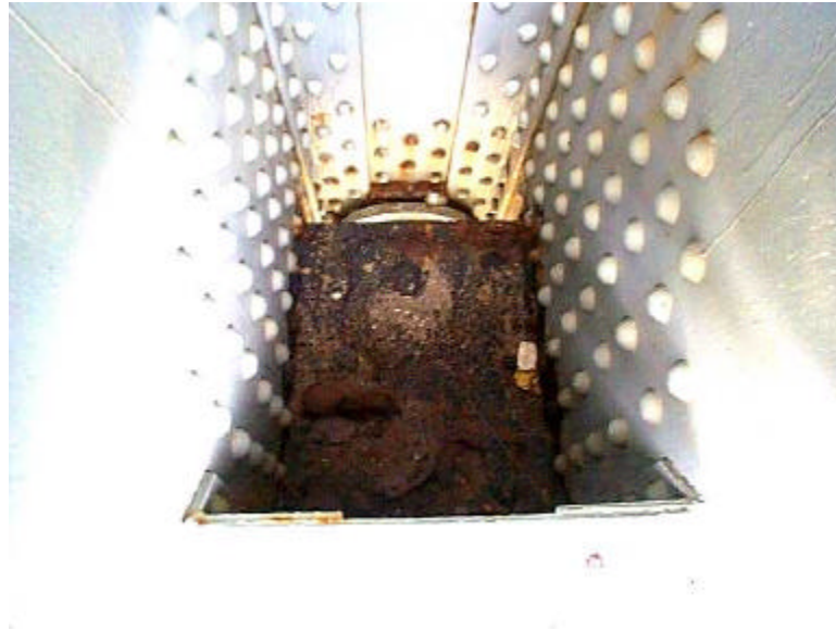
Photo 4 - Accumulation of steel shot and debris at the North Arch panel point 5'
