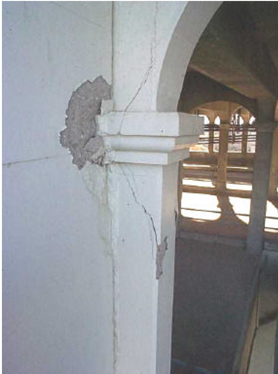
Photo 1 - Pier 12 Northwest corner spalled and cracked
