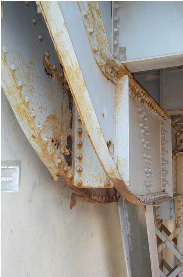
Photo 60. View showing corrosion holes in the web plates and lower flange angles at the north cantilevered end of the lower deck floor beam at Panel Point 0'.
