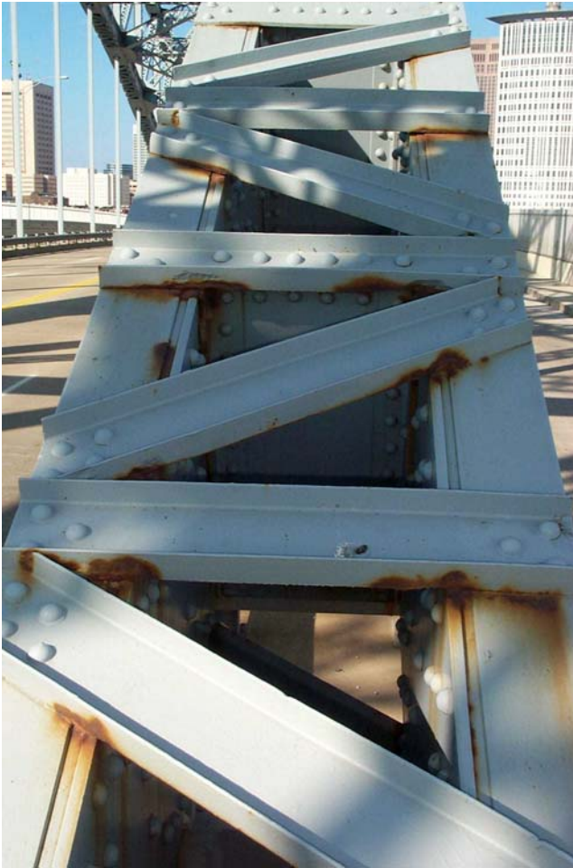
Photo 44. View looking east at areas of pitting and active corrosion on the top lacing channels of Lower Chord L5-L6 in the south truss.
