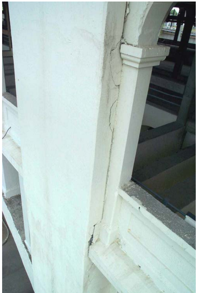
Photo 71. View of three delaminated areas on the west face of the north exterior pier shaft at Pier 8, along the interface with the upper deck column.
