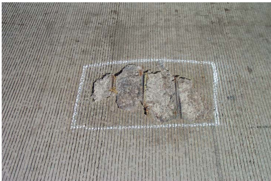
Photo 3. View showing a 20- by 30-inch spalled and delaminated area on the wearing surface in the north eastbound lane of the upper deck above East Station, at a location approximately 75 feet west of the end of the concrete wearing surface at the east end of the station.
