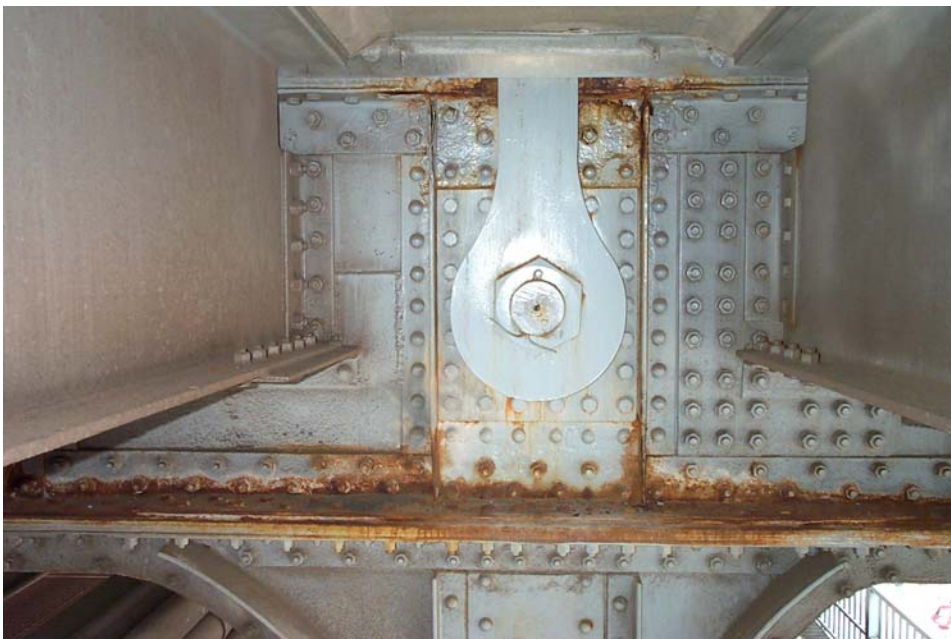
Photo 40. View from the west side of the upper deck floor beam at Panel Point 7' of the south truss. Note the corrosion that has developed on the top and bottom flange and portions of the web of the floor beam as a result of exposure to water and roadway chemicals that passed through the opening in the deck around the hanger.
