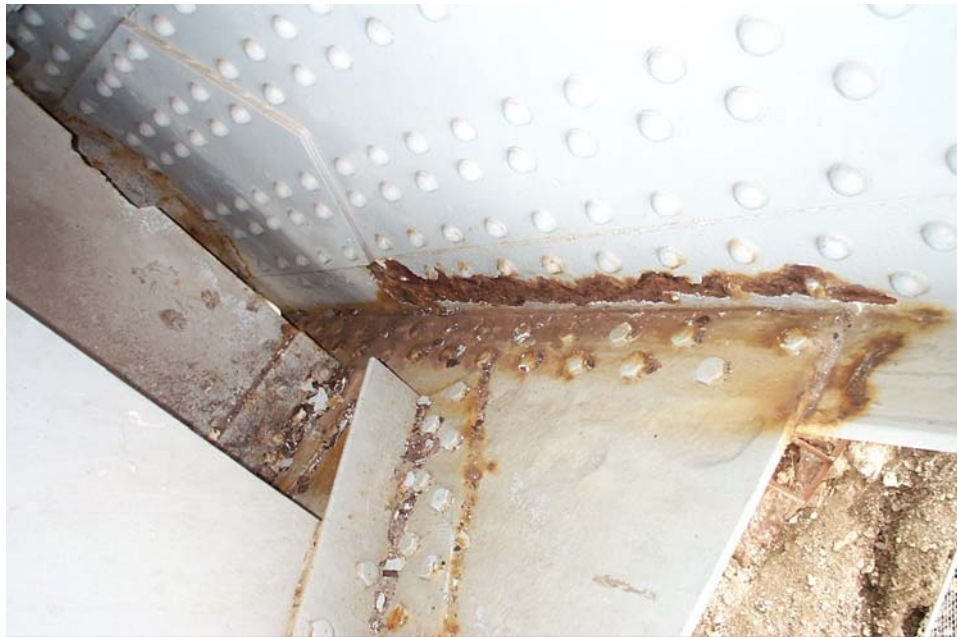
Photo 47. View showing section loss and active corrosion on the vertical leg of the lower interior angle of Lower Chord L0-L1 of the north truss adjacent to the lateral brace connection plate at Panel Point L0.
