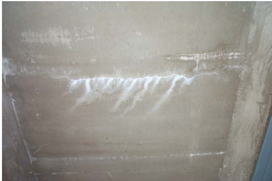
Photo 2. View showing a 0.002 to 0.003-inch wide transverse crack in the bottom side of the upper deck of Span 4 at a location between Panel Points 1' and 2' and Stringers H and J.
