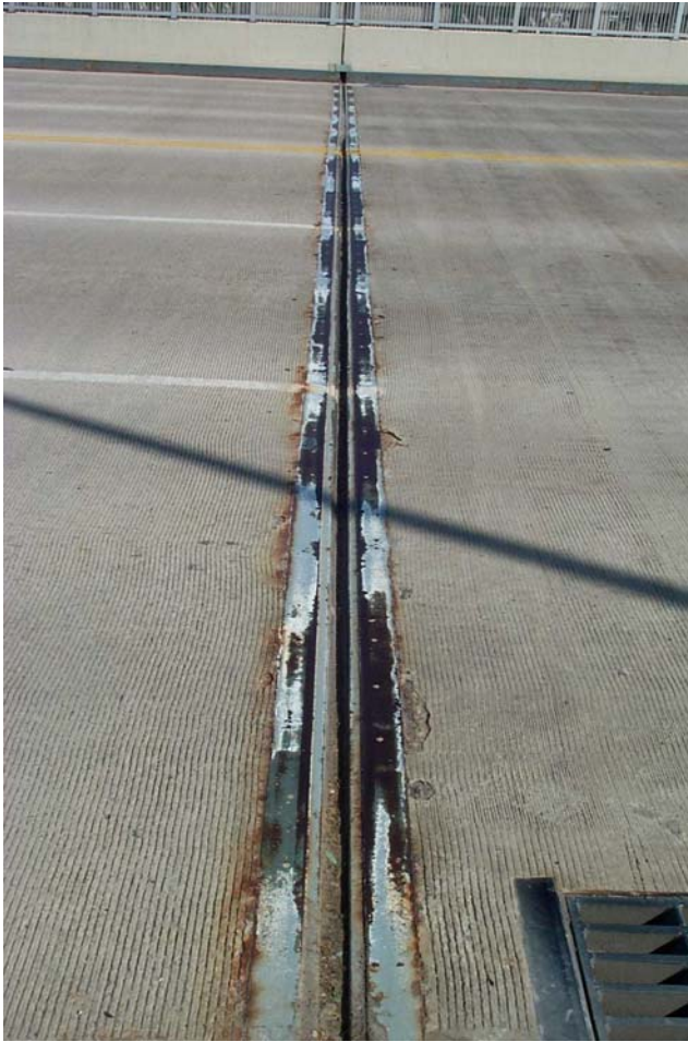
Photo 4. View looking south over the joint in the upper deck at Pier 7 showing scaled/spalled areas along the joint armor. DCP_2277.JPG
