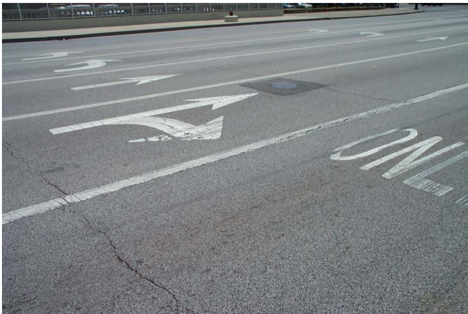
Photo 78. View looking southwestward from the west end of Span 1A showing typical transverse and longitudinal cracks in the west approach pavement.
