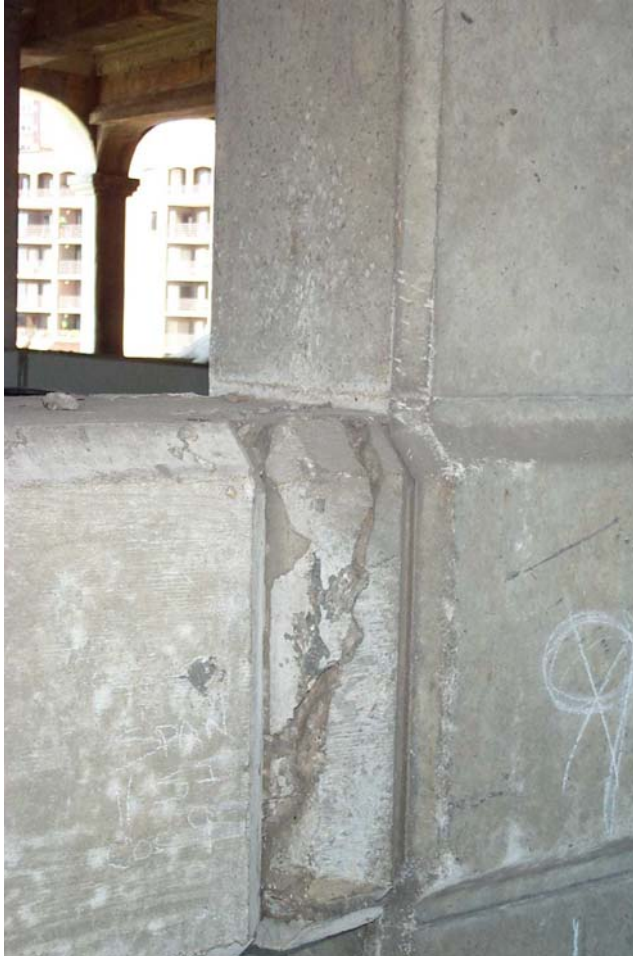
Photo 18. View of a crack through the south face of the railing adjacent to Column 1 in the south interior column row in Span 12. Note that the railing has a keyed joint at this location that coincides with the expansion joint in the deck. Insufficient opening in the key may have caused the concrete to crack from pressure encountered during movement.
