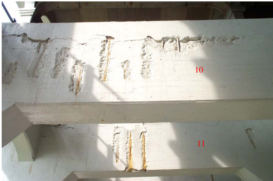
Photo 26. View looking east showing shallow spalls on the west face of Floor Beams 10 and 11 in the north bay of Span 10. Note that this condition is typical of many floor beams in Span 10 but is most pronounced at Floor Beam 10.
