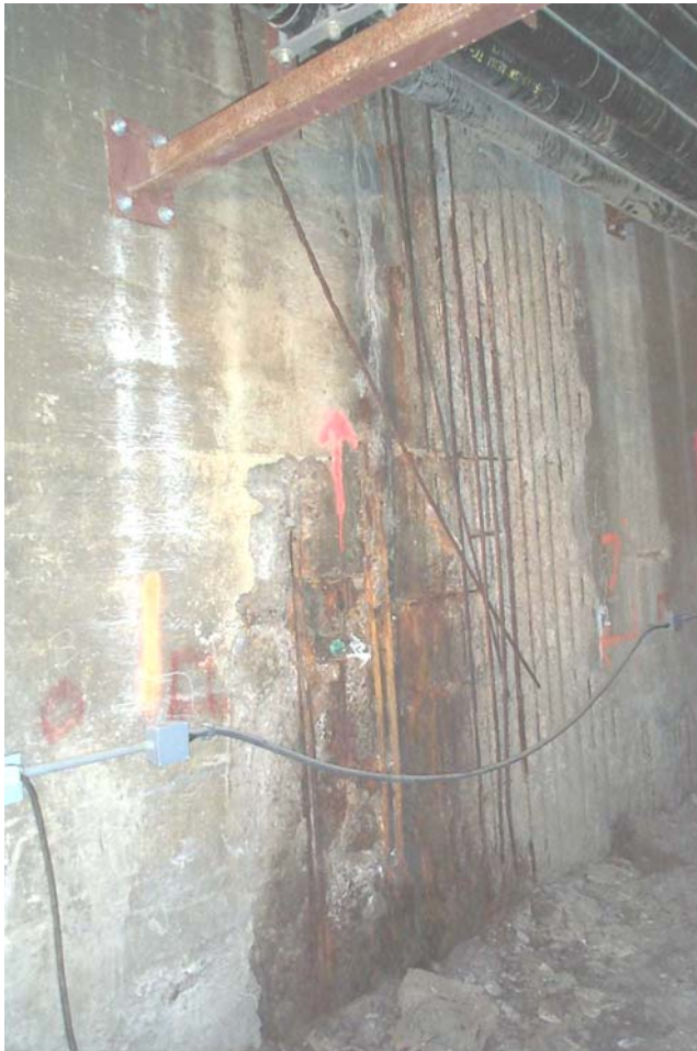
Photo 88. View of a full-height spall approximately 8 feet wide, with exposed and disbonded reinforcement. The area is located on the south wall of Detroit Avenue Subway Tunnel, below the roof slab expansion joint at the east end of the tunnel. This condition is typical at many of the expansion joints.
