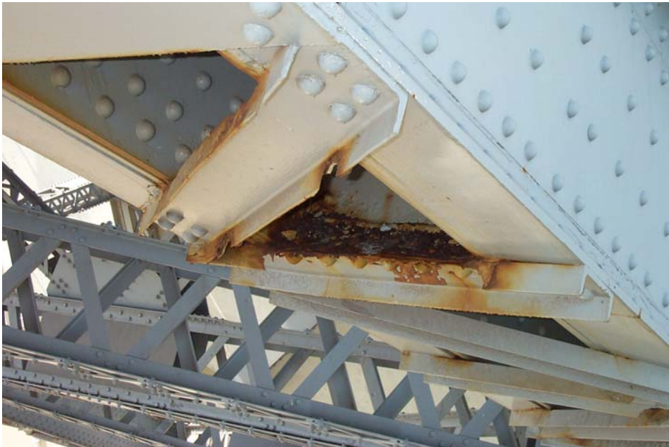
Photo 45. View of corrosion holes through the flanges of the lower lacing channels and active corrosion on the web diaphragm of the lower chord of the north truss, below Panel Point L2.
