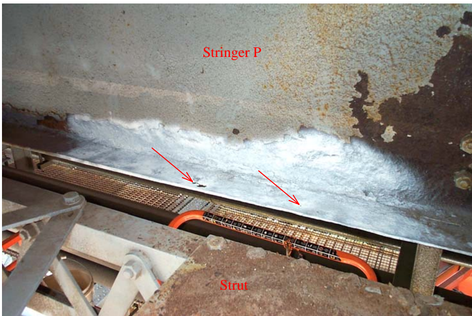
Photo 64. View from the south side of Stringer P showing a 3-foot-6-inch long area on the lower web and bottom flange where the scale was removed and white paint applied to highlight the section loss. The arrows point to a 1 x 2 1/2-inch and a 1/4-inch diameter hole in the bottom flange. The depth of pitting in the web is up to 3/8-inch. Note the close proximity of the strut member.
