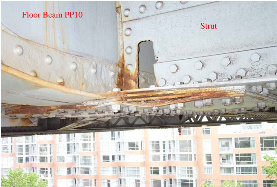
Photo 66. View from the east side of the lower deck floor beam at Panel Point 10 showing the connection to the horizontal strut located between Stringers 2 and 3. Note the pack rust between the edges of the gusset plate, fill plate, and the lower flange angles of the strut and the floor beam. Also in view is a hole coped in the web of the strut and section loss to the rivets and vertical leg of the lower flange angle of the floor beam.
