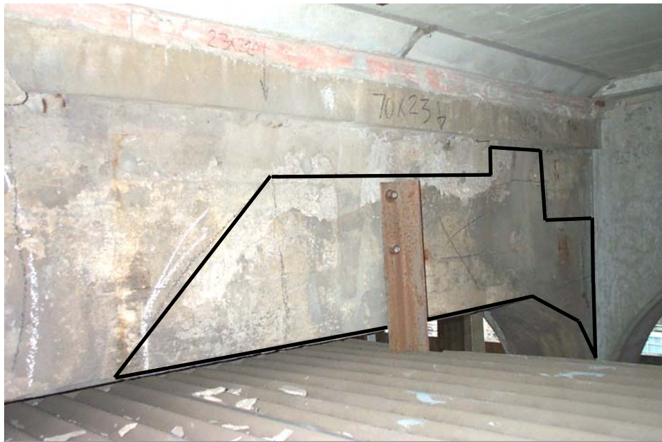
Photo 19. View of the east face of Floor Beam 15 in the south bay of Span 3. The black lines outline an area of delaminated concrete located within the north half of the beam.
