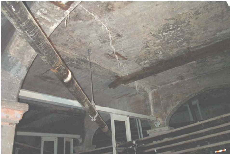
Photo 80. View looking southeastward showing a transverse crack with efflorescence and stalactites on the roof slab of West Station, between Column Rows C and D and Column Lines 7 and 8. The crack extends from the north wall to Column Row E.
