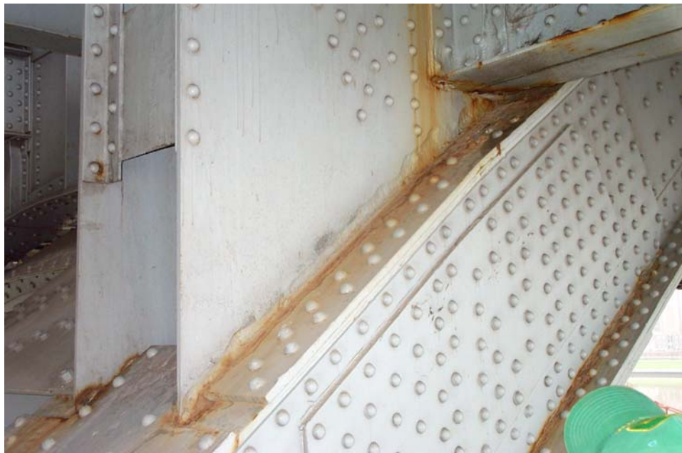
Photo 52. View of the outside face of the south gusset plate at Panel Point L3 of the south truss showing a typical band of pitting along the top plate of the lower chord.
