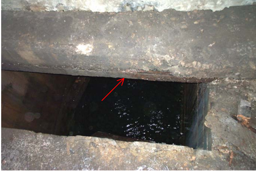
Photo 69. View inside the cellular East Abutment showing a 12- x 18-inch concrete conduit above a cell opening on the north side of the north column wall. The arrow points to the location where water is leaking from the bottom of the conduit. The type of pipe or utility that is encapsulated within the concrete is undetermined. Also in view is approximately 6 feet of water inside the cell.
