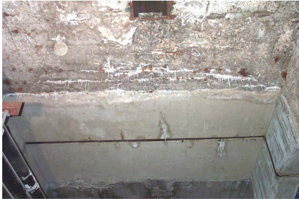
Photo 84. View looking west at the expansion joint in the roof slab between Panels 4 and 5 in the south bay of Detroit Avenue Subway Tunnel. Note the short cracks with efflorescence in the replacement concrete and the cracks, efflorescence and rust stains in the original concrete along the interface with the replacement concrete.
