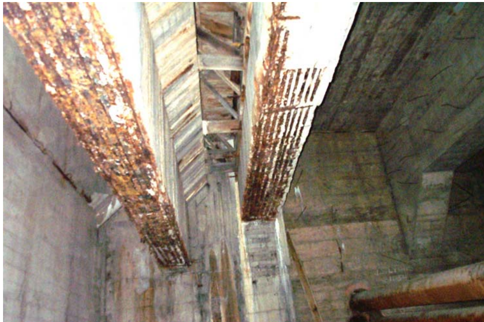
Photo 25. View looking north beneath Floor Beams 1 and 2 in the north bay inside the cellular East Abutment showing heavy spalls and corroded reinforcement along the bottom of the floor beams. The lower layer of longitudinal bars is exposed over the full length of Floor Beam 1 and the north two-thirds of Floor Beam 2 in this bay. Similar spalls expose large areas of reinforcement on these two beams in the center and south bays also.
