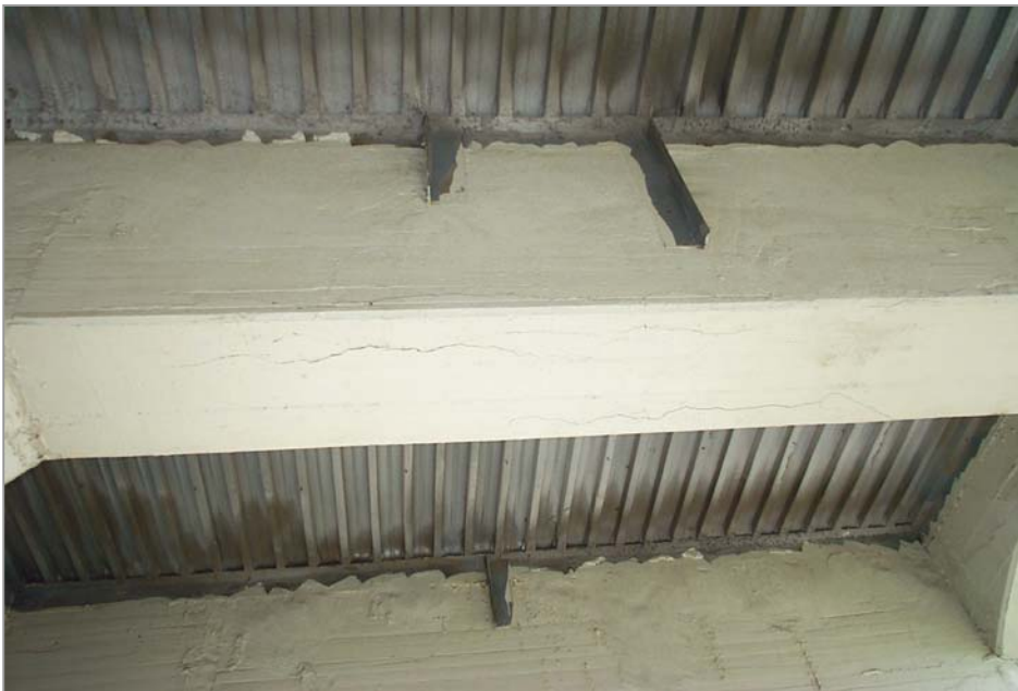
Photo 21. View looking upward showing longitudinal cracks on the bottom face and within the lower 4 inches of the west face of Floor Beam 6 in the south bay of Span 3. A similar crack is present within the lower 4 inches of the east face also. The concrete below the cracks in the vertical faces and on the entire bottom face is delaminated.
