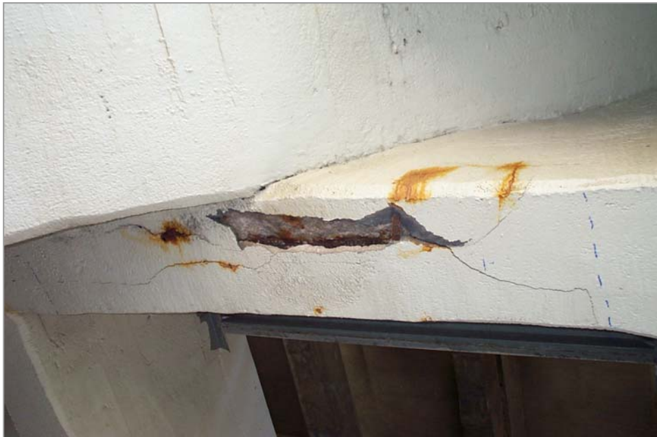
Photo 24. View showing a delaminated and spalled area on the bottom face of the longitudinal beam adjacent to the north exterior arch ring that connects the ends of Floor Beams 10, 11, and 12 in Span 12. Note that this area lies directly above a parking lot and that the concrete is separated and loose.
