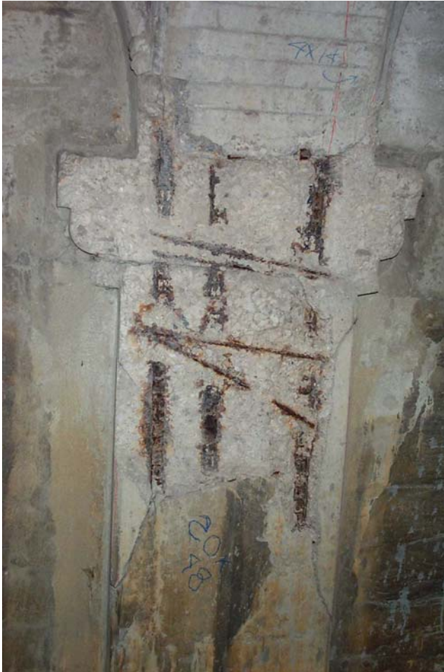
Photo 30. View showing a spalled area on the south face at the top of Column 6 in the north central column row in Span 1A. Note that the south protrusion of the corbel detail has fallen away and the spalled area extends the full width of the column and up to 48 inches down from the top.
