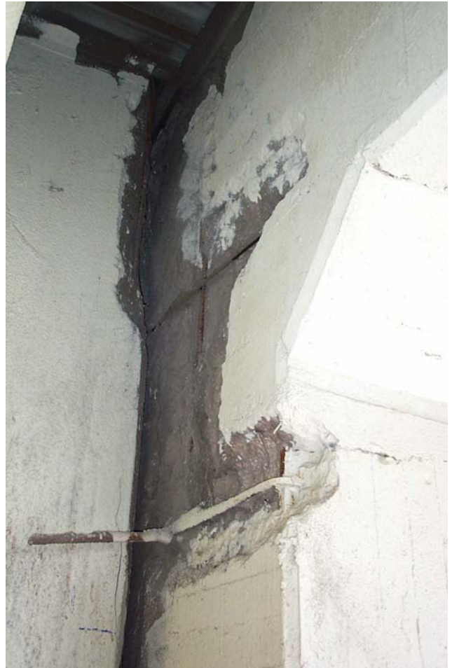
Photo 33. View showing 36- x 42-inch and 36- x 36-inch spalls on the west face and a 6- x 8-inch spall on the south face of Column 1 in the south interior row in Span 6.
