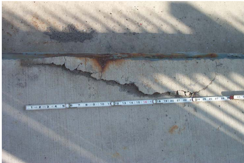
Photo 6. View showing a 28-inch long by up to 6-inch wide delaminated and spalled area on the north sidewalk along the curb plate in Span 13.
