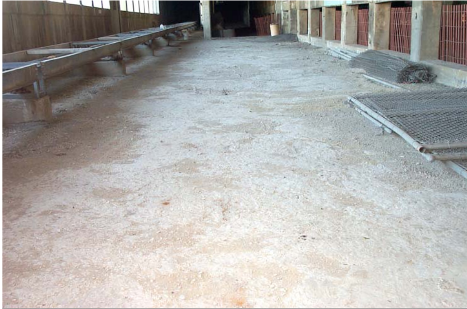
Photo 17. View looking west through the south bay of Span 1B showing the poor condition of the surface of the original lower level concrete deck.
