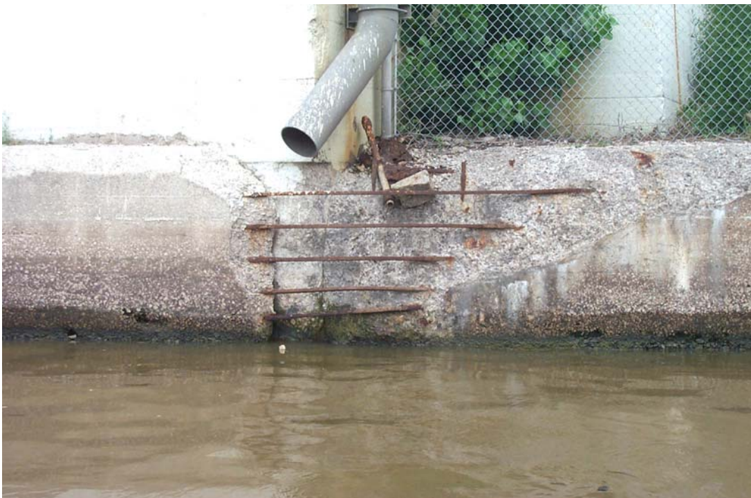
Photo 4. View looking northeastward showing the large spalled area on the concrete cap of the protection wall along Pier 4. The area is approximately 12 feet wide at the top of the cap and tapers to a width of approximately 2 to 3 feet below the water surface and exposes a total of 8 horizontal reinforcement bars (see Pier No. 4 Plan View, Sheet 11).
