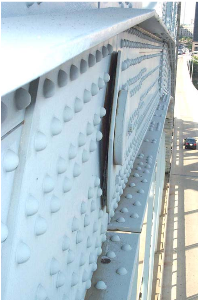
Photo 43. View looking east along the south side of the lower chord at Panel Point L12 of the south truss showing a gap between the web of the chord and the edge of the cover plate caused by the expansion of pack rust behind the plate.
