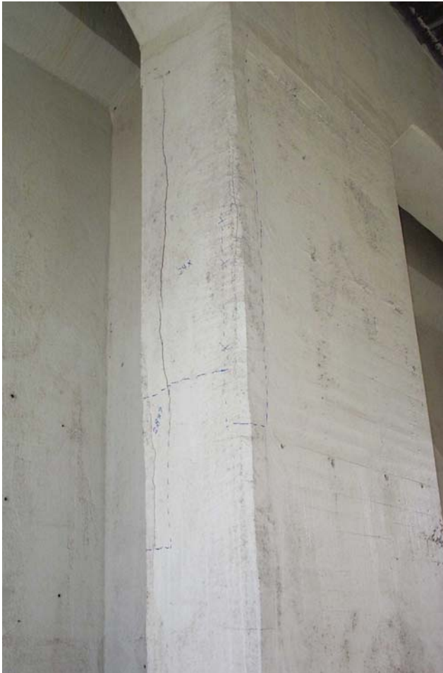
Photo 32. View showing areas of delamination outlined by blue lines on the south and east faces and a longitudinal crack along the west edge of the south face of Column 1 in the south interior row in Span 8. A total of 31.9 square feet of delaminated concrete was recorded for this column.
