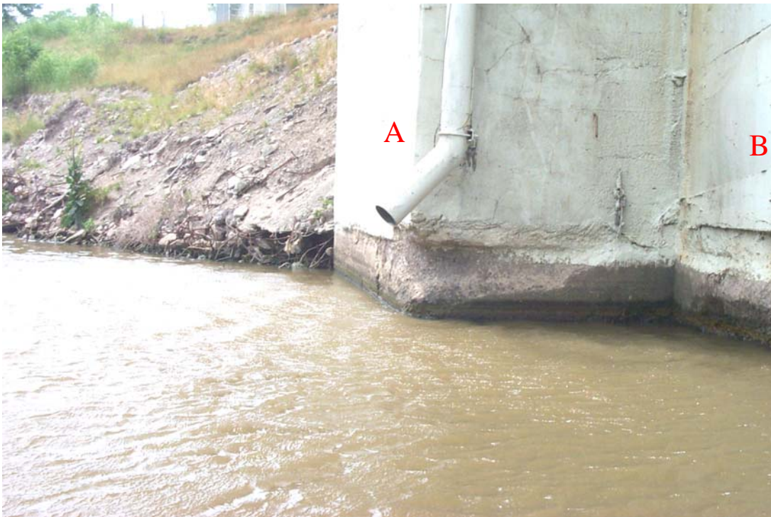
Photo 2. Additional view looking west showing the spalled and missing concrete within the splash zone at corners A and B of Pier 3. This condition does not appear to have changed significantly from what was reported in the previous inspection.
