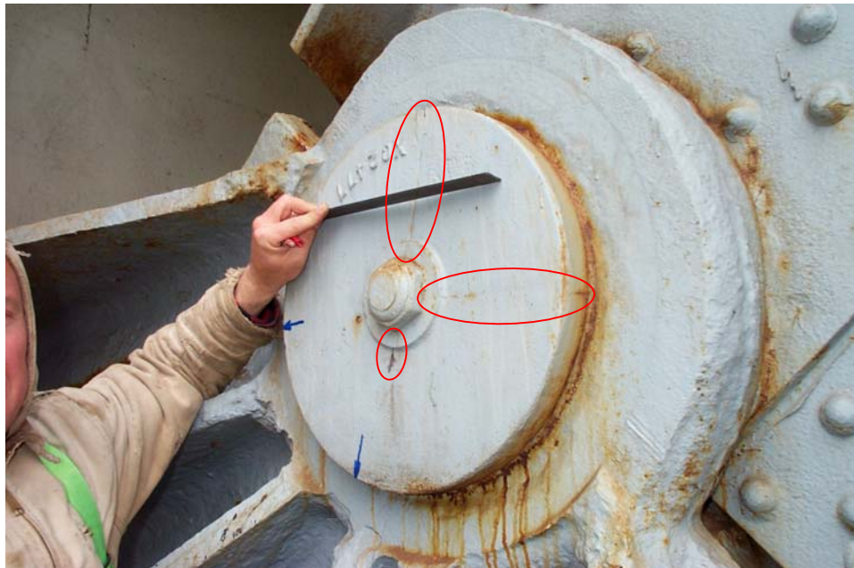
Photo 68. View showing radial and edge cracks (ovals) in the face of the retaining washer on the south side of the bearing at the west end of the south arch rib. The straight edge shows cupping in the face of the washer at the upper crack. The arrows point to the locations of transverse cracks at the edge of the washer. Note the active rust that shows at the interface of the washer and the flange of the shoe.
