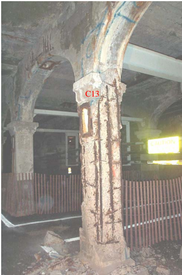
Photo 82. View looking southeastward showing deep spalls with exposed and disbonded reinforcement on the north and west faces of Column C13 in West Station. Similar spalls are present on half of the south face and portions of the east face of the column. Also in view are spalls with exposed reinforcement and surrounding delaminations on the north and bottom faces of the adjacent jack-arch beam.
