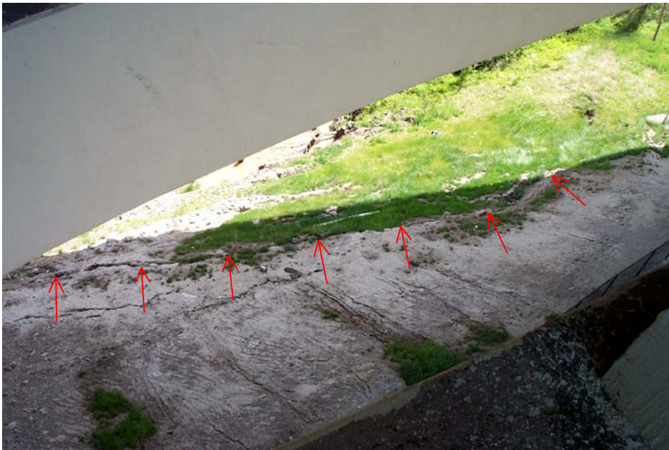
Photo 76. View looking south showing the area of slope failure in the embankment west of Pier 3. The arrows point to the cracks formed where the embankment has separated. Note that the cracks are partially obscured by the grass.
