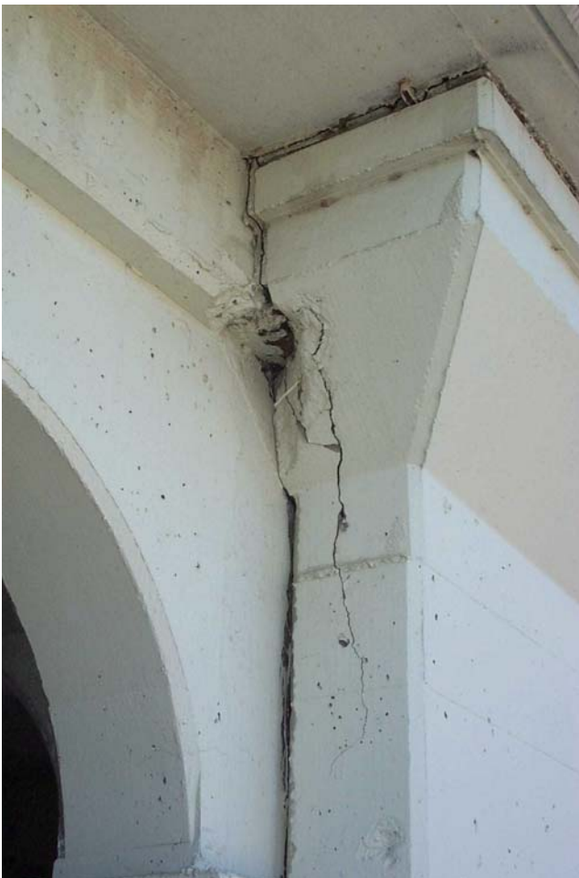
Photo 70. View of a 10- x 50-inch spall/delamination on the east face of the north exterior pier shaft at Pier 1, just below the sidewalk at the upper level deck.
