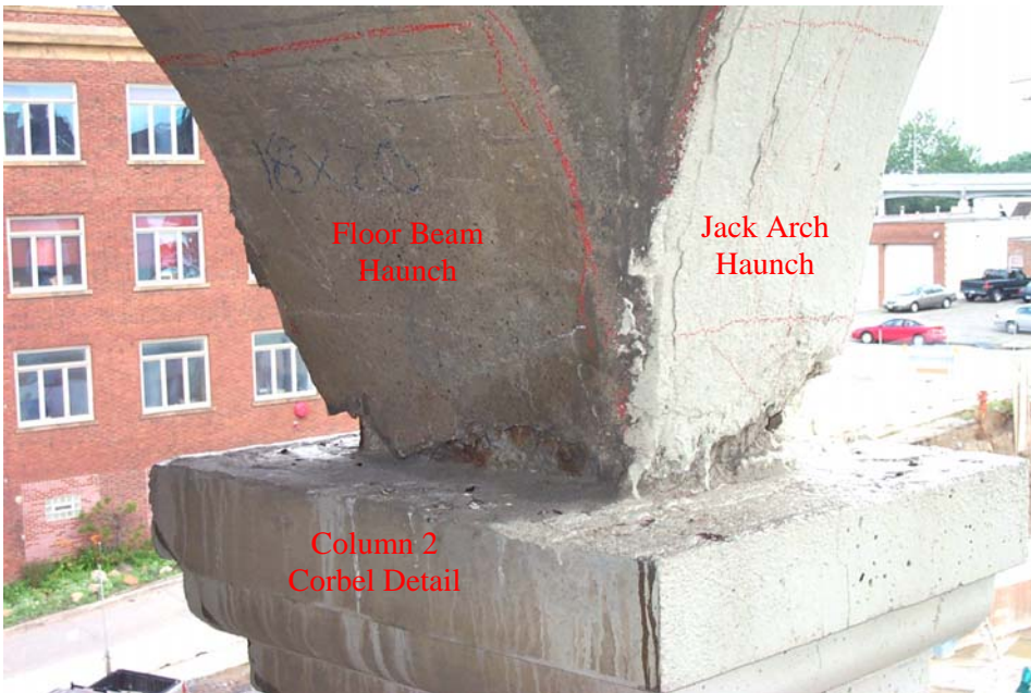
Photo 28. View of the corbel detail at the top of Column 2 in the north exterior column row in Span 2. The red lines outline areas of delaminated concrete on the bottom face at the base of the floor beam haunch and the jack arch haunch. Also in view are spalled or void areas along the haunch interface with the top of the corbel detail.
