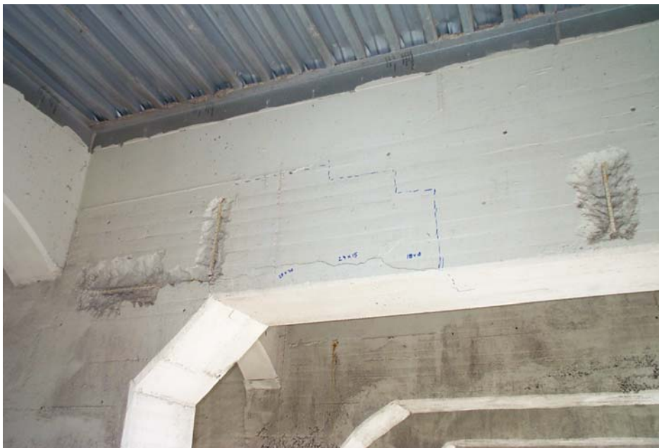
Photo 22. View of the bottom and west faces of Floor Beam 2 in the south bay of Span 5. The blue dashed lines show the edges of an area of delaminated concrete that extends to the right of the spalls above the spandrel column. Note that the concrete on the bottom face of the floor beam below the marked area is also delaminated.
