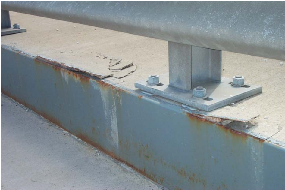
Photo 7. View showing 9½-inch wide by 30-inch long and 4-inch wide by 10½-inch long spalled and delaminated areas along the north curb plate of the north arch-truss island between PP7 and PP8. Also in view are areas of rust along the top and bottom of the curb plate. DCP_2282.JPG
