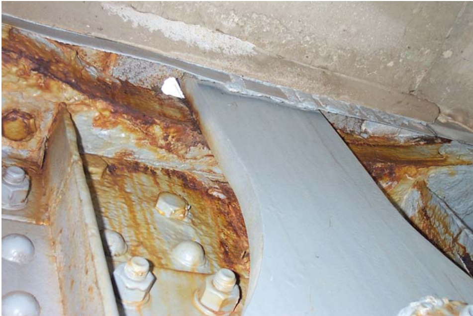
Photo 39. View of the opening through the deck around the west eyebar hanger for the upper deck floor beam at Panel Point 8 of the north truss. Note the active corrosion on the web and top flange of the floor beam. The corrosion on the opposite face of the hanger is hidden from view.
