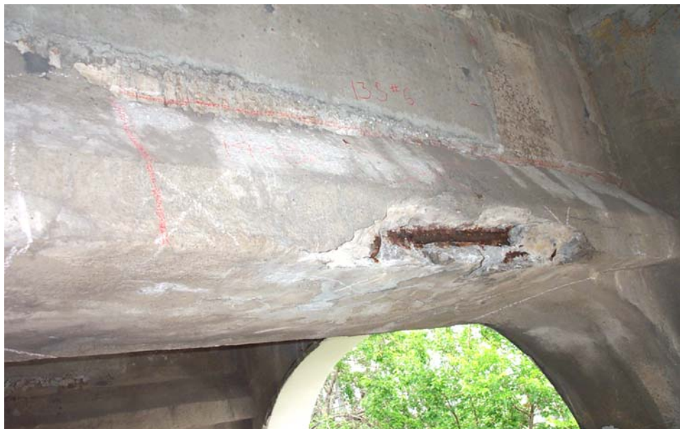
Photo 20. View of the lower portion of the west face and the bottom of Floor Beam 6 in the south bay of Span 13 showing a spall with exposed reinforcement. The widened section at the bottom of the beam encapsulates extra reinforcement added at the end portions of the original beams during the 1967 rehabilitation as a strengthening measure. The red lines outline delaminated concrete that was part of the strengthening repair. Areas of delamination are fairly typical at the strengthened beam ends.
