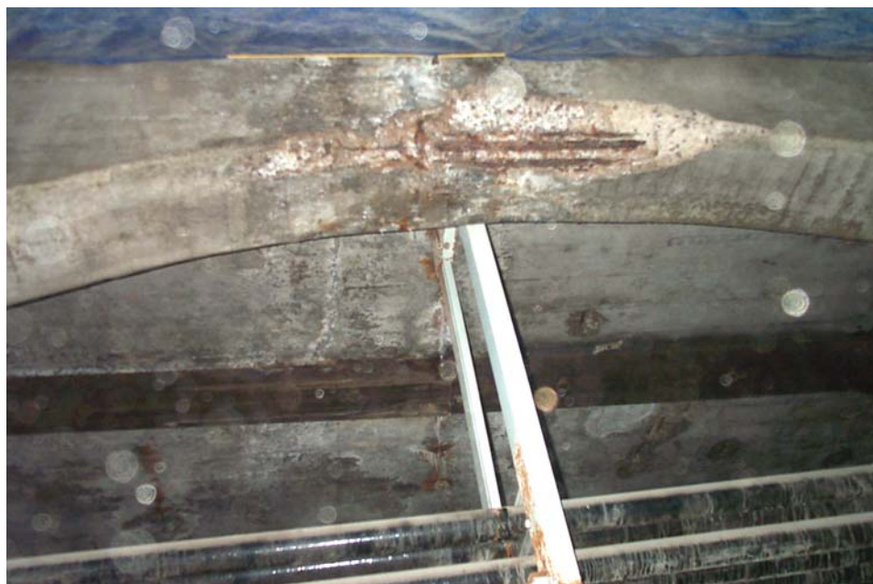
Photo 85. View looking south showing spalls with exposed reinforcement on the north and bottom faces of the jack-arch beam located between Columns 7 and 8 in Detroit Avenue Subway Tunnel. Also in view is a typical transverse crack with efflorescence on the roof slab in the south bay.
