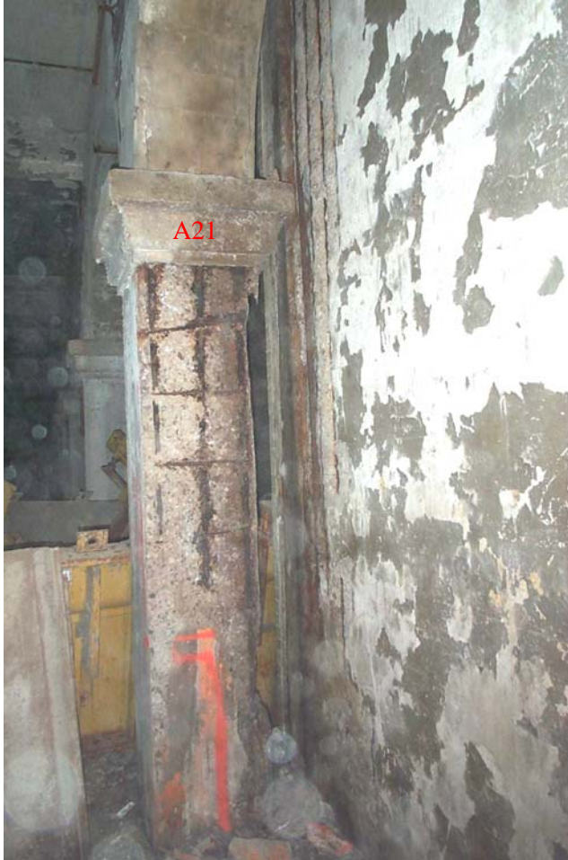
Photo 83. View looking west showing deep spalls with exposed reinforcement on the east face of Column A21 in West Station. Similar deterioration was noted on the west face and a portion of the north face of the column. Also in view is a spalled area several feet wide that extends over the full height of the north wall.
