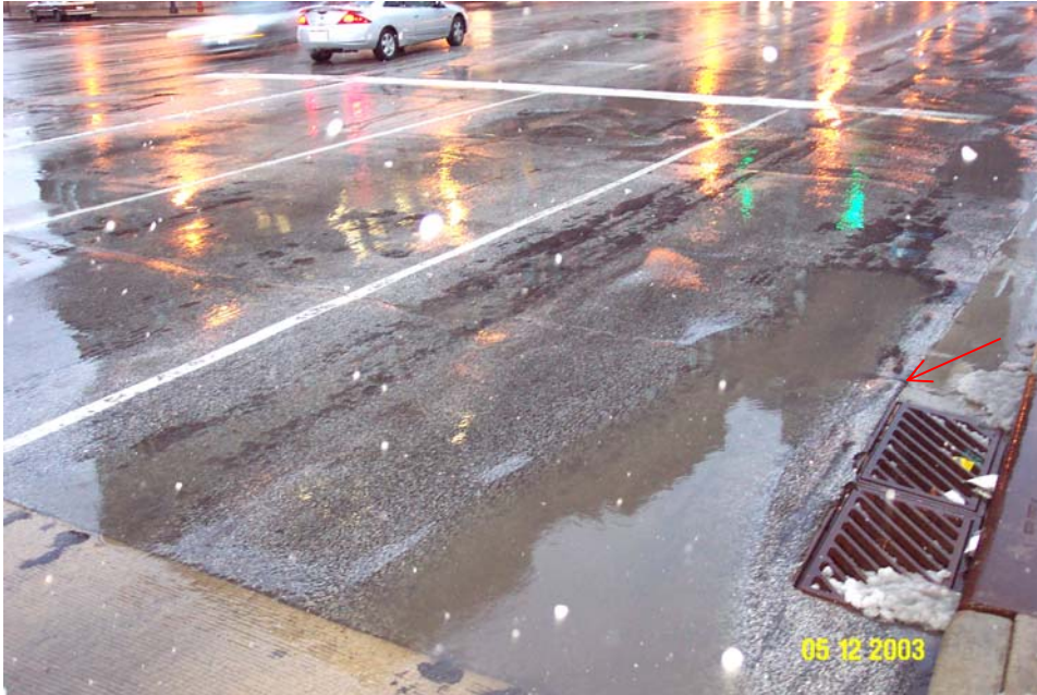
Photo 77. View looking northeastward from the end of the concrete wearing surface, showing the condition of the asphalt pavement in the eastbound lanes of the east approach. Note the wheel line grooves in the south and center lanes and the wide transverse crack (arrow) that extends across the entire roadway.
