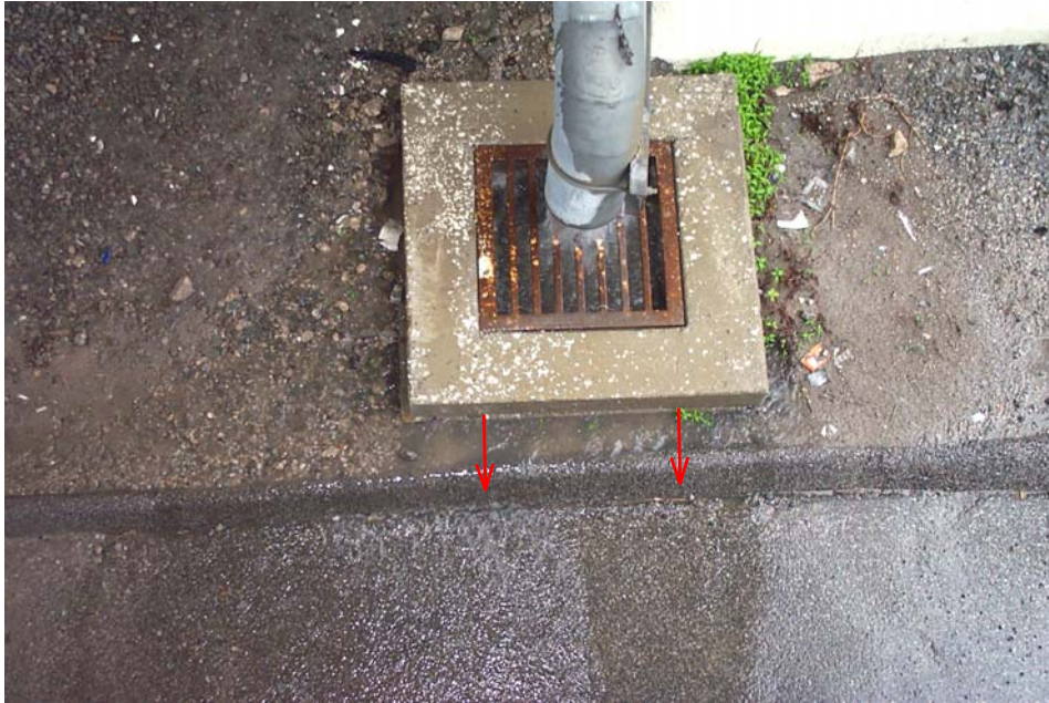
Photo 12. View looking down at the downspout and catch basin at Pier 9 South showing water leaking under the lid of the basin (arrows) and flowing into the adjacent parking lot. DCP_2375.JPG
