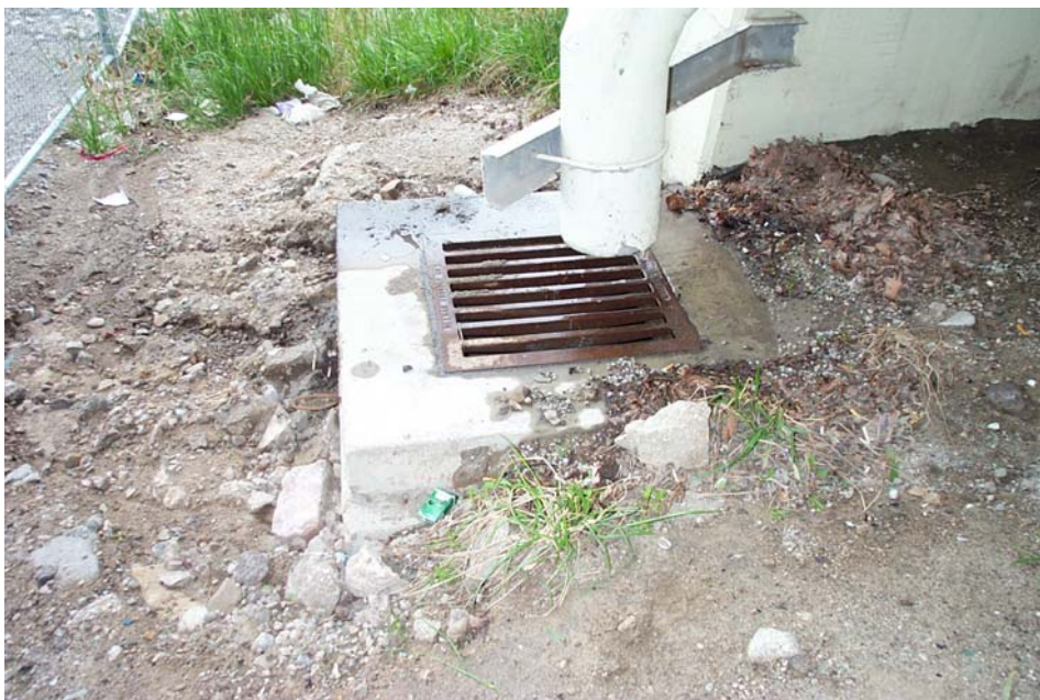
Photo 9. View looking south showing the end of the downspout and the lid of the catch basin at Pier 1 South. Note that the lid could be moved up to 5 inches to the north, which would better align the spout with the grate.
