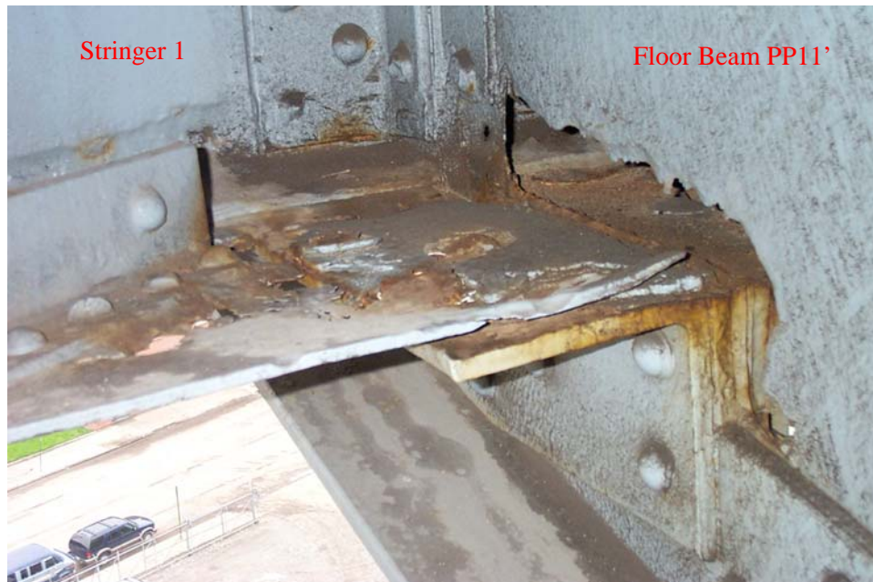
Photo 62. View from the east side of the lower deck floor beam at Panel Point 11' showing a typical corrosion hole through the web, above the north half of the seat angle at Stringer 1. Also in view are perforations through the connection plate, and groove pitting and a 1-inch diameter hole in the lower web of the stringer.
