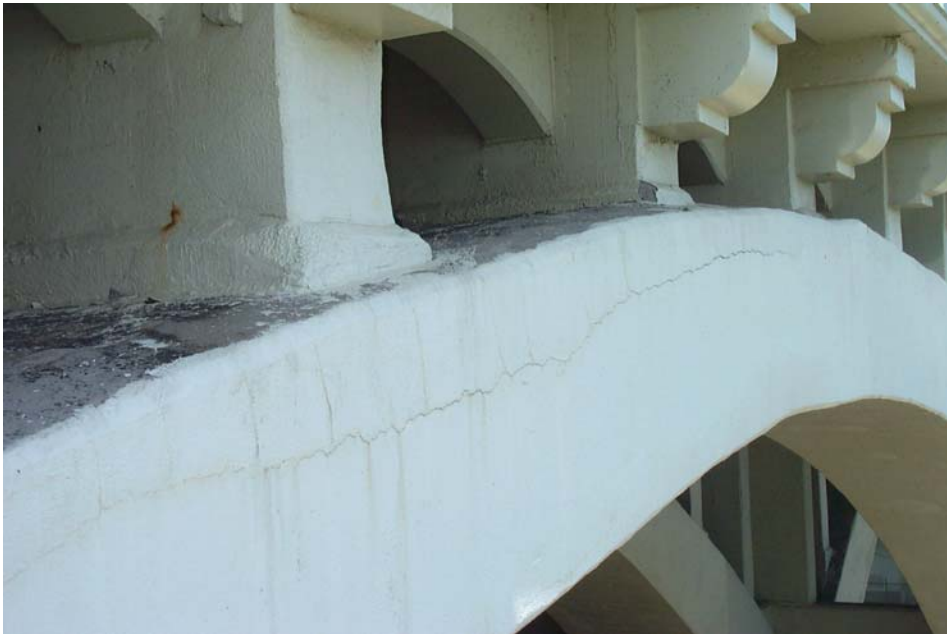
Photo 34. View showing a concentric crack located approximately 12 to 16 inches below the top of the south face of the south exterior arch rib, that extends from the 3 rd to the 6 th spandrel column bay in Span 1. Note that the concrete within the area above the crack is patch concrete and is delaminated. Also, a similar size area of delaminated patch concrete is present along the adjacent edge of the top face of the rib.
