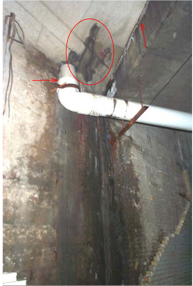
Photo 11. View looking southeastward showing the PVC downspout below the deck scupper in the south gutter at the east end of East Station. The horizontal arrow points to the junction where water escapes through the gap between the vertical spout and the elbow. The oval highlights the area where water is leaking through holes drilled into the deck floor. Also note the water leaking through the adjacent deck joint (vertical arrow).
