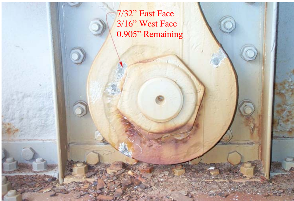
Photo 56. View of a circular band of pitting on the outside face of the east hanger, at the connection to the lower floor beam at Panel Point 4 of the south truss. The pitted area is approx. 1 1/2 to 2 inches wide and extends between the positions of 7 and 11 o'clock (moving clockwise). A similar area of pitting is present on the opposite (inside) face of the hanger and extends between the positions of 3 and 2 o'clock (moving clockwise). The measurements show the depth of pitting and remaining bar thickness at the location measured. Also note the pieces of heavy rust scale lying on the beam flange that were removed from the inside face of the hanger to determine the depth of section loss. DCP_2476.JPG
