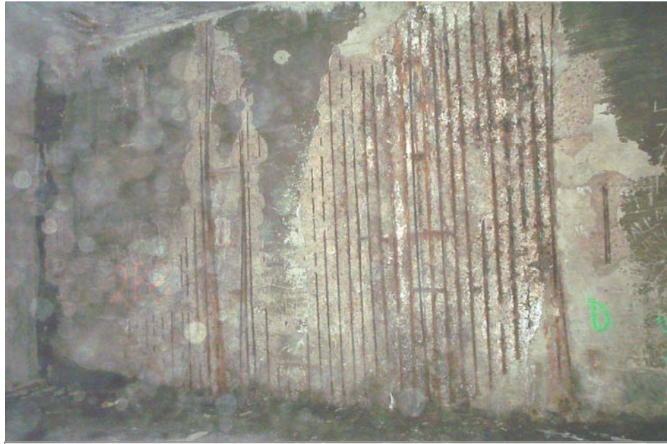
Photo 87. View of the north wall of Detroit Avenue Subway Tunnel in an area adjacent to Columns 1, 2 and 3 showing large full-height spalls with exposed and disbonded reinforcement. The tunnel closure wall is visible at the left of the photo.
