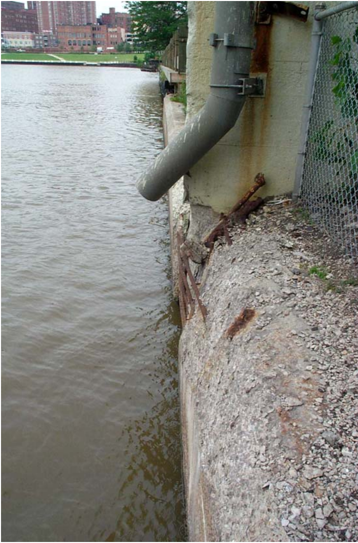
Photo 5. Additional view looking downstream along the concrete cap of the protection wall showing the spalled area on the cap adjacent to the corner of Pier 4.
