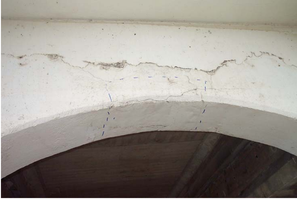
Photo 27. View looking north showing the jack arch between Columns 9 and 10 in the south exterior column row of Span 5. The dashed blue lines highlight the edges of an area of delaminated concrete on the south and bottom faces.
