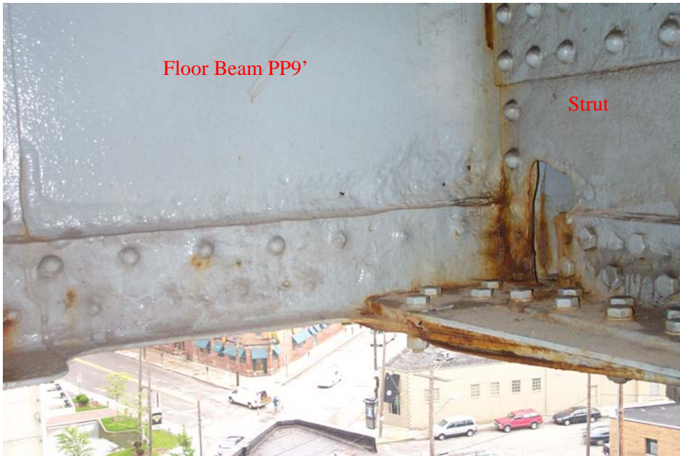
Photo 63. View from the west side of the lower deck floor beam at Panel Point 9', on the north side of the connection to the strut located between Stringer Lines 2 and 3. Note the band of deep pitting and perforations in the floor beam web along the lower flange angle, the section loss to the angle, and the portion of the lower flange that has been coped. Also note the coped hole in the web of the strut and the reactivated corrosion.
