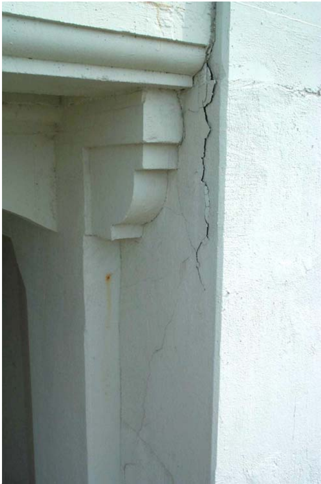
Photo 72. View of a delaminated area on the east face of the north exterior pier shaft at Pier 6, adjacent to the corbel detail at the top of the spandrel column.
