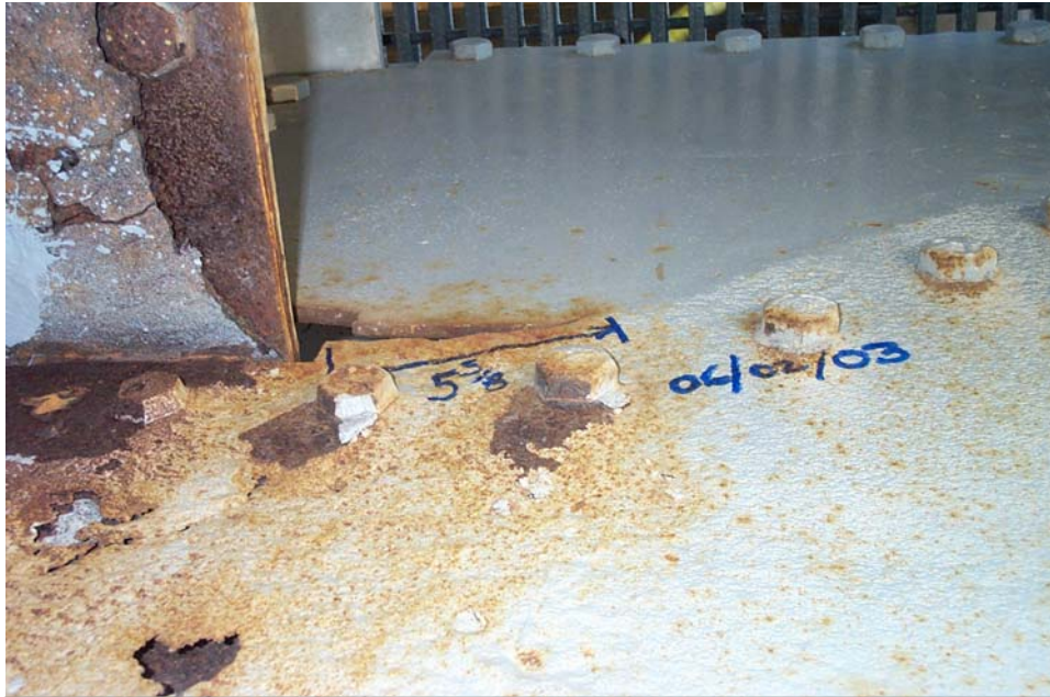
Photo 61. View showing a 5 5/8-inch long crack in the west web plate of the lower deck floor beam at Panel Point 0, adjacent to the north edge of the lower flange of Stringer 12. Not in view are large corrosion holes in the floor beam web below the stringer.
