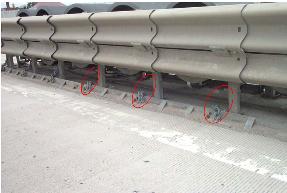
Photo 8. View from the south side of the LMA device located at the west end of the south arch truss. The ovals show locations where the anchor chain is disconnected from the horizontal pin on the leg of the LMA device. DCP_2642.JPG
