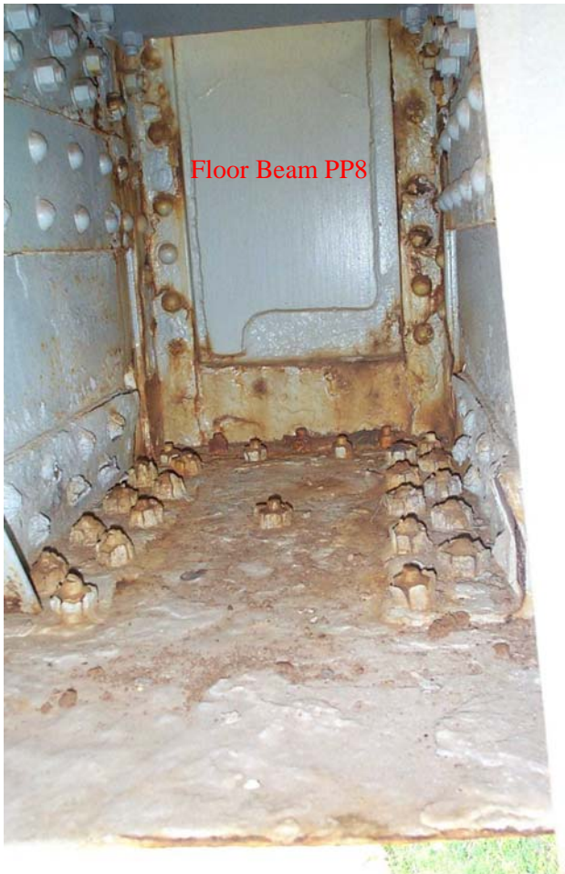
Photo 67. View inside the horizontal strut between Stringers 10 and 11, looking towards the connection on the east side of the lower deck floor beam at Panel Point 8, showing areas of flake rust that were painted over at the time of the last rehabilitation.
