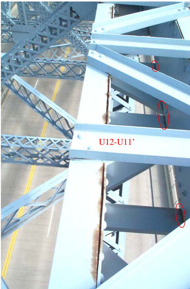
Photo 42. View looking east along Top Chord U12-U11' of the south truss showing areas of initial pack rust and active corrosion between the top edge of the north web plate and the vertical leg of the angle. The ovals highlight areas where the corrosion has reactivated on the web of the lower lacing channels. DCP_2512.JPG
