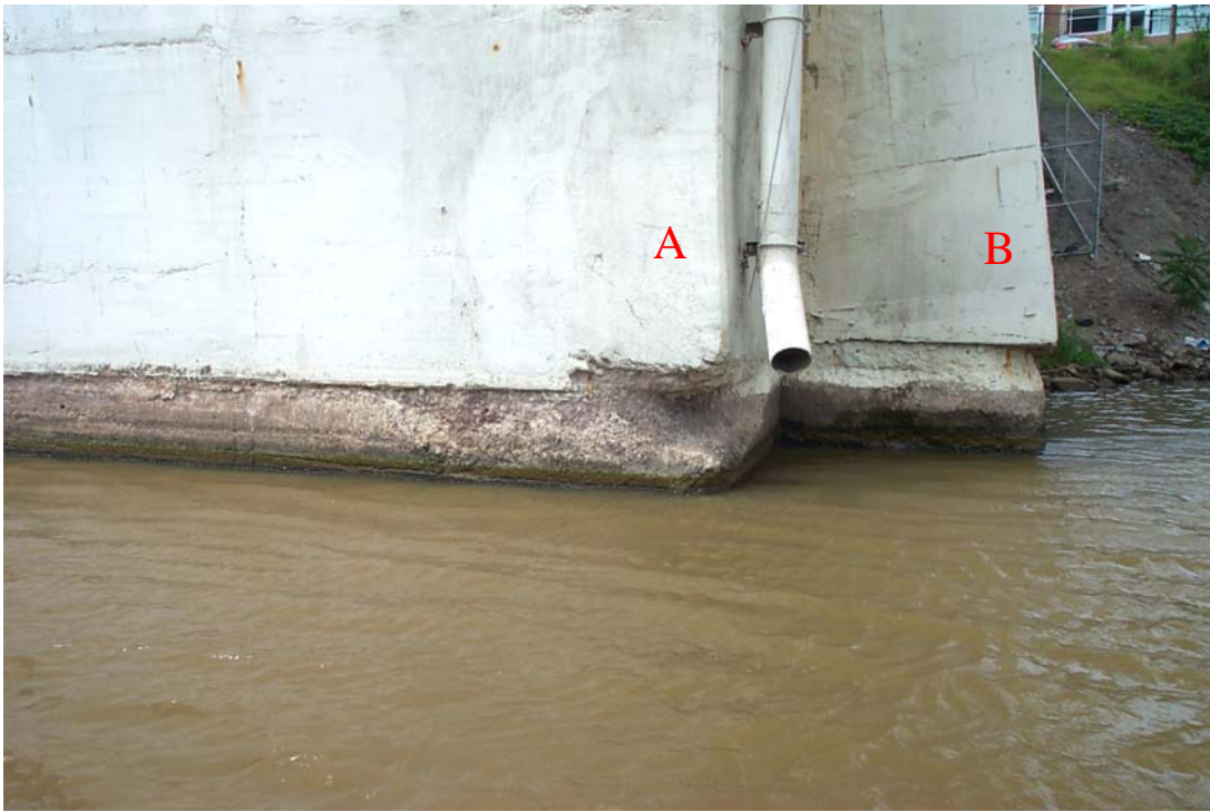
Photo 1. View looking northwestward showing deterioration of the concrete of Pier 3 in the splash zone between the water line and a horizontal construction joint or lower limit line of former concrete repair. Note the rounding at the corners marked “A” and “B” where the concrete loss ranges from 16 to 24 inches in depth. Loss of section in other areas within the splash zone varies up to 6 inches in depth. Not visible in the photo are spalled or dished-out areas at corners A and B below the water line with concrete loss extending 3 to 6 inches into the pier, and rounding at the corners with concrete loss of up to 9 inches (see Pier No. 3 Plan View, Page 9 and Pier No. 3 Detail A and B, Page 10).
