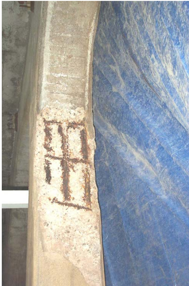
Photo 86. View looking west showing a large spall with exposed reinforcement on the east face within the upper half of Column 44 in Detroit Avenue Subway Tunnel. County maintenance workers performing repairs to the north wall erected the blue tarp along the column line.
