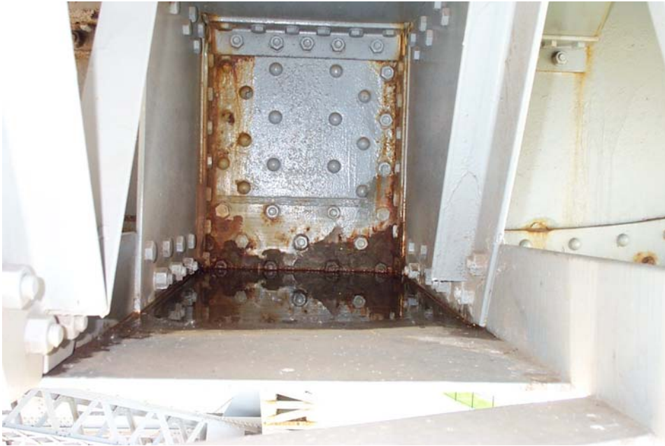
Photo 41. View looking west through the horizontal strut at the connection to the lower deck floor beam at Panel Point 4 of the north truss showing corrosion on the web of the floor beam and water collected inside the strut. The water, which originates from above the upper deck, flows down the vertical and accumulates in the connection area. DCP_2347.JPG
