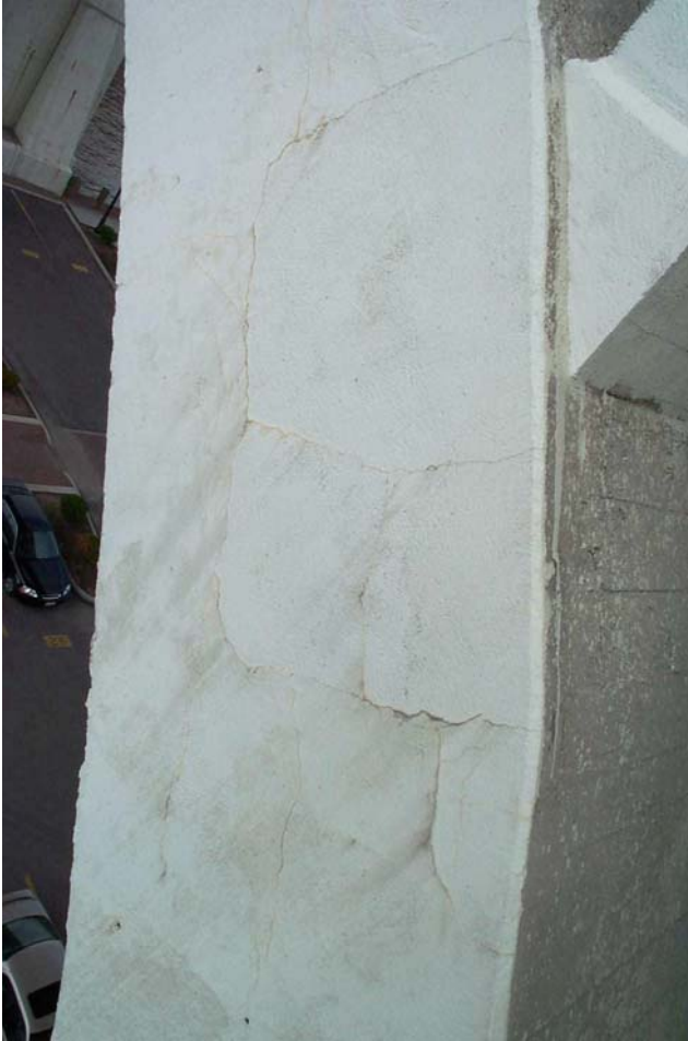
Photo 36. View showing map cracks on the south face of the south arch rib near the 14 th spandrel column in Span 5. No delaminations were detected by sounding in this area.
