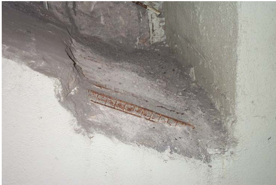
Photo 37. View showing reinforcement exposed in a 22- x 36-inch area on the top surface of the north interior arch rib in Span 13, adjacent to East Abutment. This area appears to be what remains of a larger area that was prepared for patching, which was not completed.
