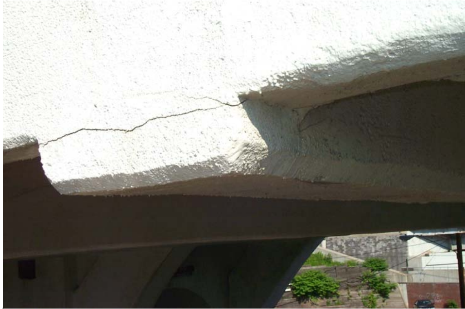
Photo 23. View showing a horizontal crack in the north end face of Floor Beam 5 in Span 12, approximately 5 inches above the bottom of the beam. The crack separates an area of delaminated concrete that extends 9 inches inward (south) along both vertical faces of the floor beam and 19 inches on the bottom face. A similar crack and area of delamination was noted at the ends of several other beams in Span 12.
