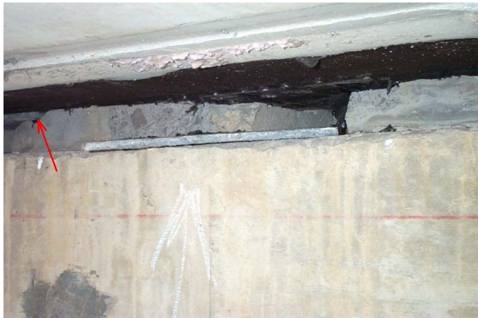
Photo 16. View showing an 11- x 9- x 3/8-inch plate that has slid from its original position between the deck floor and the pedestal on the floor beam in the center bay below the deck joint at Pier 11. The red arrow points to the front edge of the adjacent plate that is in its intended position.
