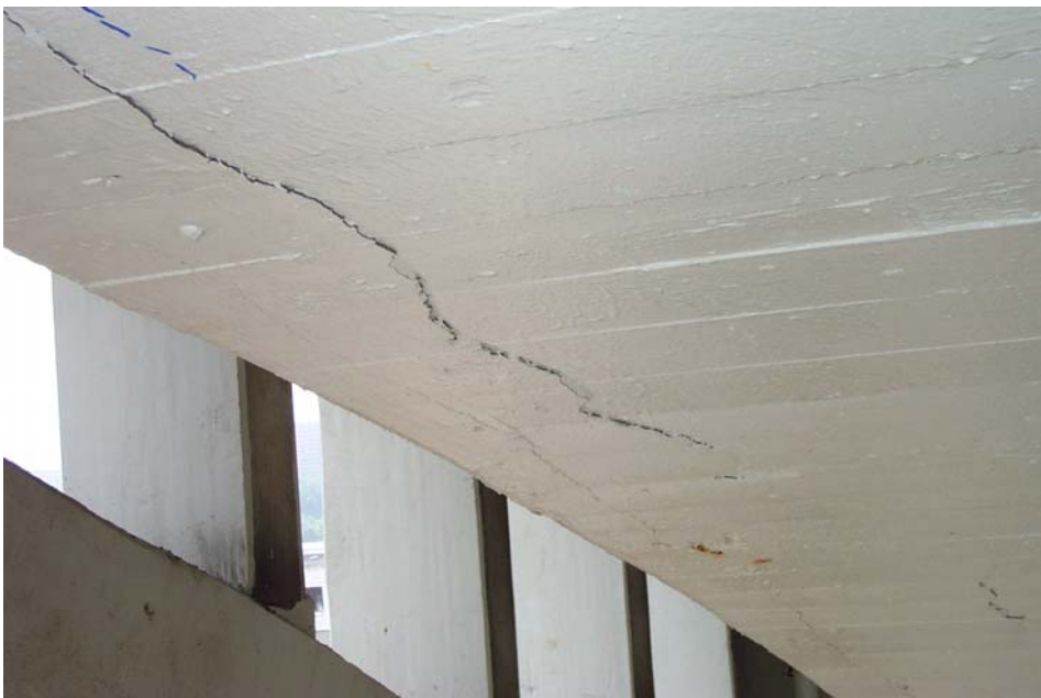
Photo 35. View showing a 13 to 20-inch wide delaminated area of original concrete along the south edge of the bottom face of the south interior arch rib below the 6 th spandrel column bay in Span 7. This band of delaminated concrete extends below the next two spandrel column bays to the west and is positioned above West Avenue.
