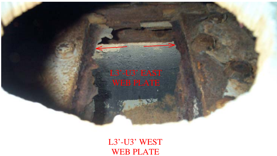
Photo 59. View looking through a 7-inch wide hole cut in the west web plate of Vertical Post L3'-U3' of the south truss, showing a portion of the web of the upper deck floor beam enclosed within the vertical post. The arrows point to the vertical edges of an 8-inch wide hole corroded through the web plate of the floor beam (between vertical stiffener angles). The hole extends vertically through the top half of the web, and the lower half is heavily scaled and thin in this area.
