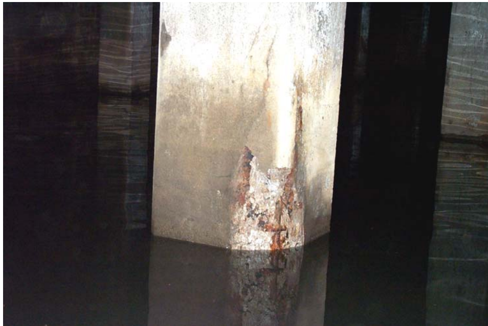
Photo 79. View showing a spalled and delaminated area at the corner of the south and west faces at the bottom of Column 22 in Column Row N in East Subway Tunnel. The spalled area extends to the floor of the tunnel that was covered by a pool of water 8 inches deep at this location at the time of the inspection.
