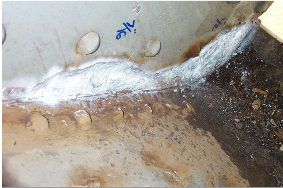
Photo 46. View inside Lower Chord L2-L3 of the south truss at the first diaphragm east of Panel Point L2. The white paint highlights an area of scale on the inside face of the north inside web plate, along the web diaphragm. The measurements show the depth of section loss where the scale was removed. Note that the scale was not removed from the entire area.
