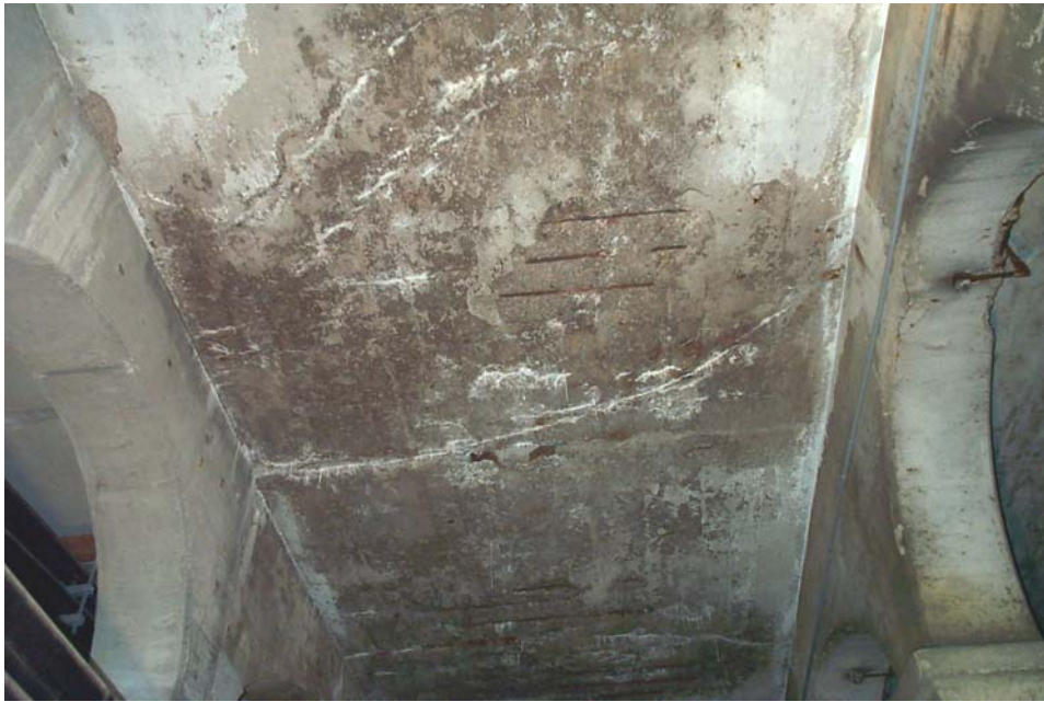
Photo 81. View looking west showing spalls and transverse cracks with efflorescence on the roof slab of West Station, between Column Rows C and D and Column Lines 29 through 31.
