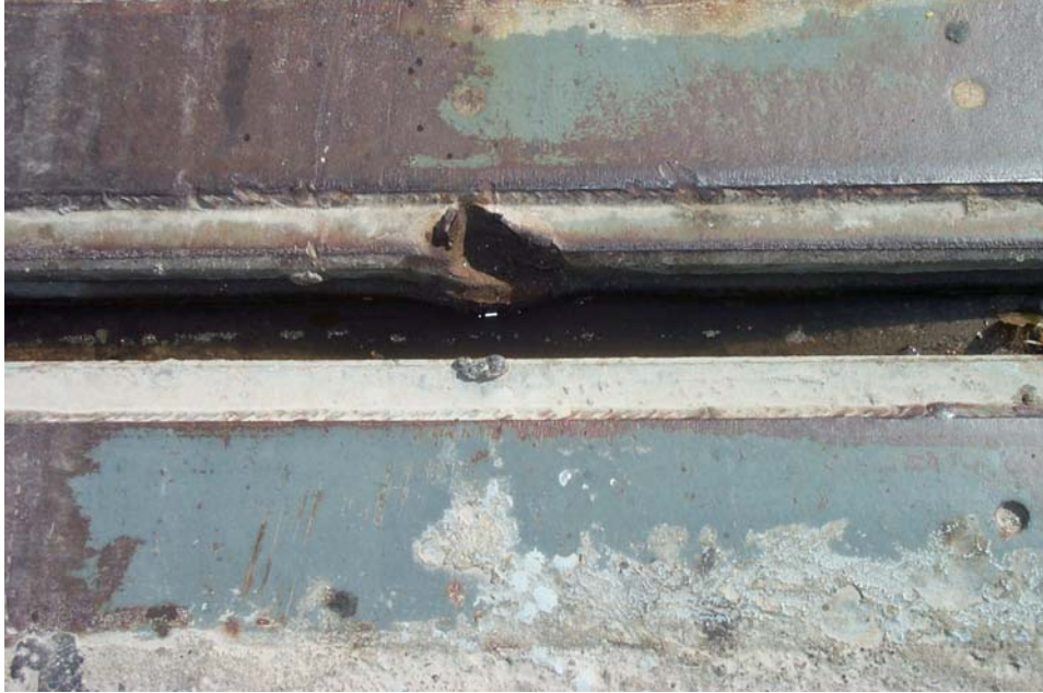
Photo 14. View showing a 2-inch long tear in the joint armor on the east side of the east joint at Pier 3, near the center of the south eastbound lane.
