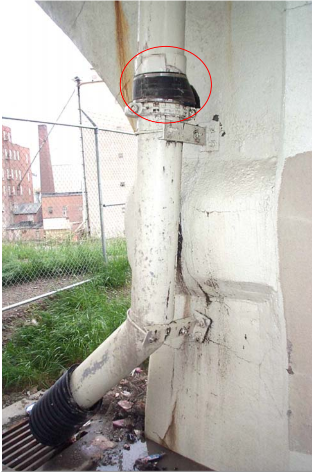
Photo 10. View looking southeastward showing the broken connection collar and rubber repair strip (oval) and the CPP extension at the bottom of the downspout at Pier 2 South. Note the water pooled alongside the pier that leaked out of the collar.
