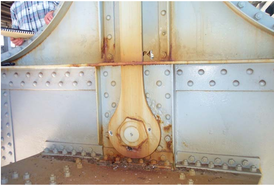
Photo 49. View from the east side of the connection bracket above the lower deck floor beam at Panel Point L4 of the north truss showing pitted areas and holes in the vertical plate of the bracket. Also note the deep pits and holes corroded through the web stiffener plate of the floor beam, adjacent to the pin.
