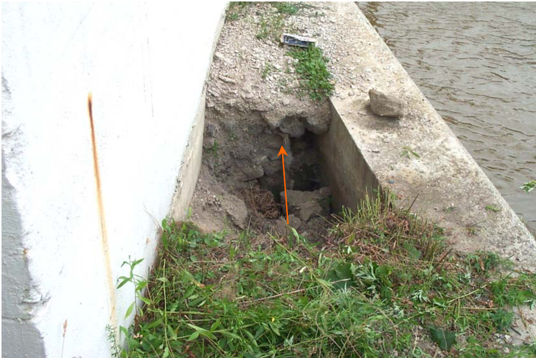
Photo 3. View looking southeastward showing the hole eroded in the embankment between the concrete cap of the protection wall and the downstream face of Pier 4. The embankment is moving in the direction shown by the arrow through a vertical gap that exists between the sheet piling supporting the cap and the face of the pier (see Pier No. 4 Plan View, Sheet 11).
