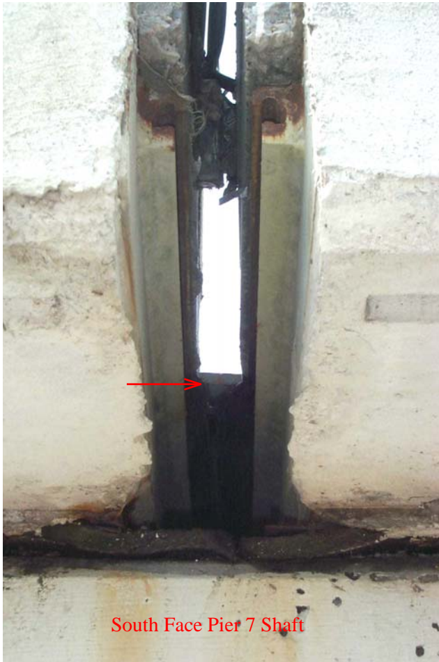
Photo 15. View looking north beneath the sidewalk overhang at the south end of the deck joint at Pier 7. Note that the end of the elastomeric gland (arrow) stops 2 inches short of the south face of the pier shaft and 13 inches short of the end of the joint armor.
