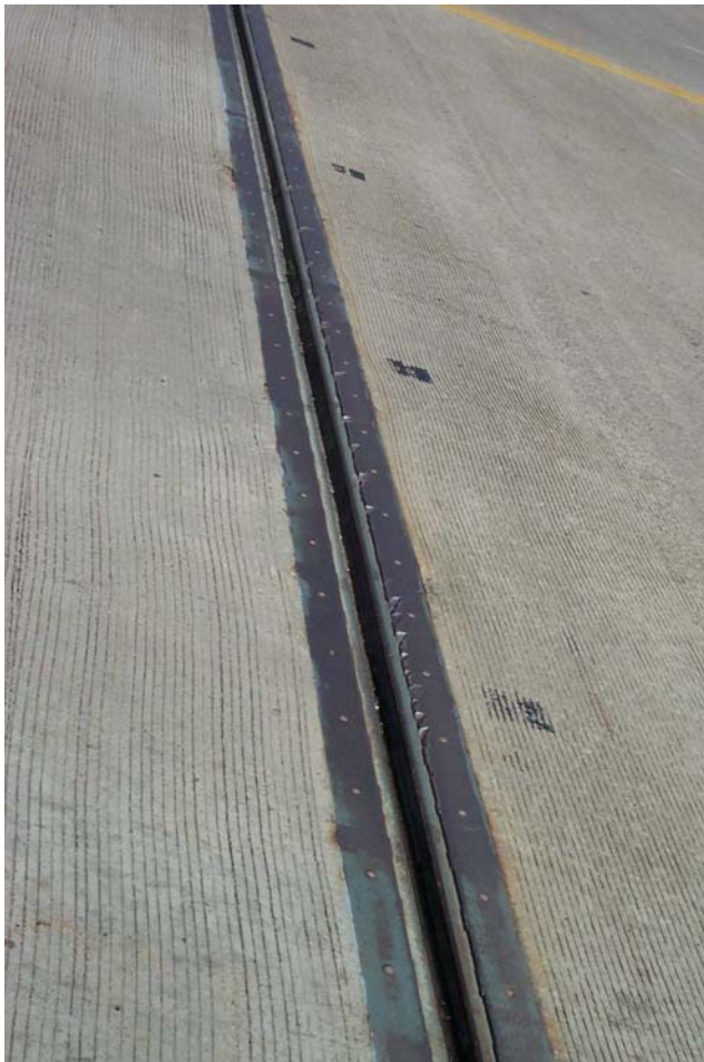
Photo 13. View looking south showing gouges in the joint armor along the west side of the deck joint at Tower B. Also note the absence of paint and light rust on the armor. DCP_2276.JPG
