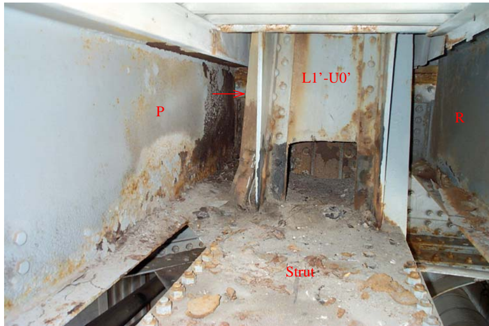
Photo 51. View looking east between Stringers P and R towards the intersection of the horizontal strut with Diagonal L1'-U0' of the south truss, showing accumulations of blasting material and areas of rust that were either painted over or missed. Not visible in the photo are the rust and scale that remain on the surfaces inside and on the north side of (arrow) the diagonal, extending from the horizontal strut up to the connection to Vertical Post L0'-U0'.
