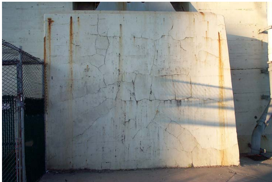
Photo 75. View of the west face of the pedestal for the south truss at Pier 4 showing map cracks and rust stains.
