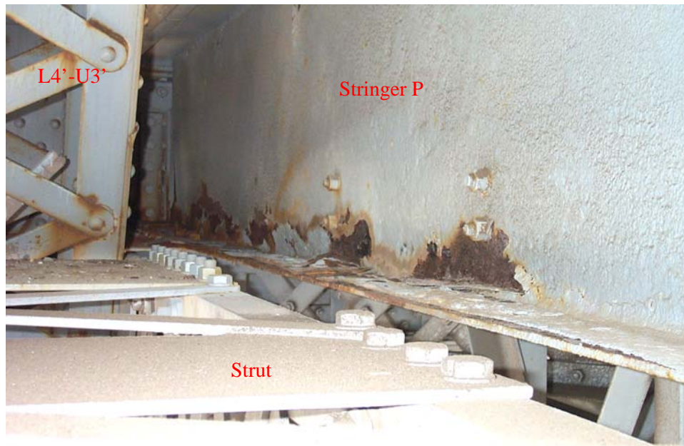
Photo 65. View looking west along the south side of Stringer P, between Panel Points 3' and 4', showing heavy scale on the lower web and bottom flange. Note that the web has a few perforations in this area and the flange is thinned to 3/16-inch at a few locations.
