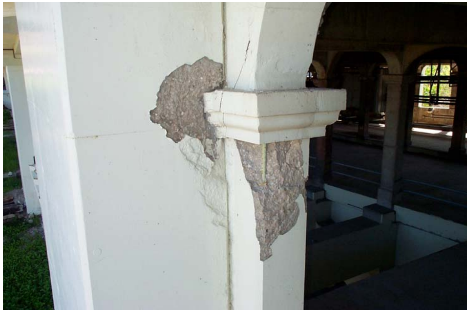
Photo 31. View showing a spalled area on the west and north faces at the top of Column 12 in the north exterior column row in Span 12. Note that portions of the corbel detail and the jack arch are cracked and delaminated in this area. The epoxy coating on the exposed reinforcement bar indicates that the column was replaced in the 1995 rehabilitation and thus the concrete deterioration developed in a short period of time. Also in view is a spall on the west face of the pier shaft. The east sidewalk along Robert Lockwood, Jr. Blvd. passes directly below this location.
