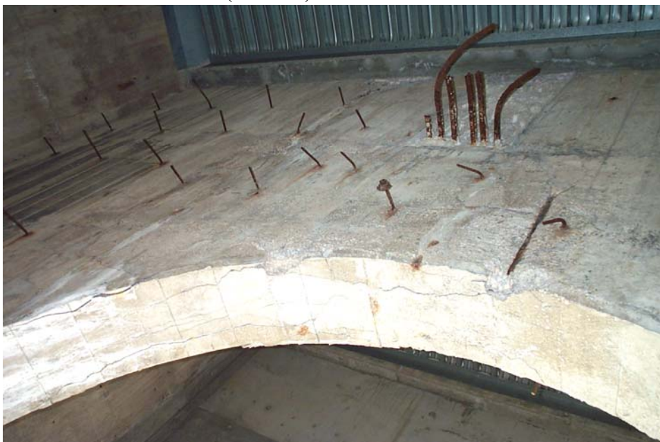
Photo 74. View inside the north bay of the tower at Pier 4 showing cracks, delaminations and spalls on the bottom and west faces of the jack-arch beam.
